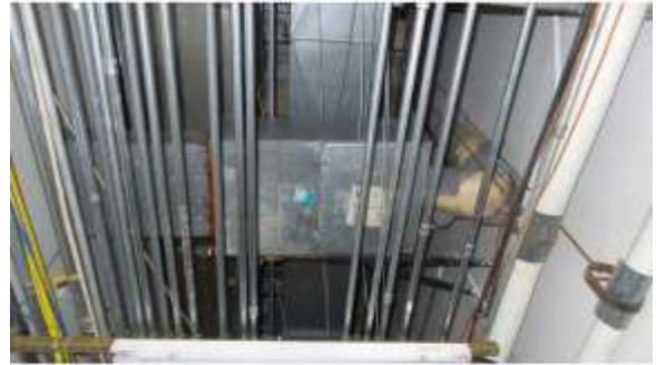
BROD046e 4/19/2016 Original variable air volume terminal box Room 8S08B
