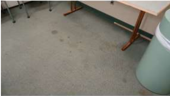
BROD044a 4/19/2016 Stained carpet Third floor
