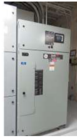
BROD097e 4/19/2016 Automatic transfer switch Generator building
