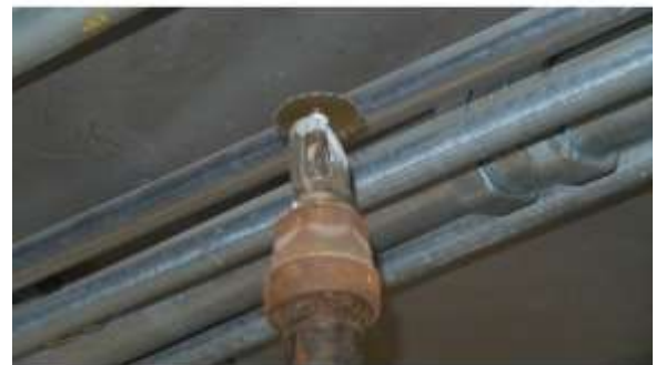
BROD039e 4/19/2016 Original fire system sprinkler head Room 8S09
