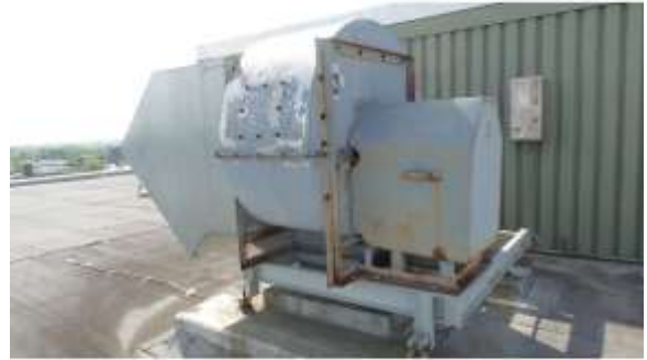
BROD004e 4/19/2016 Utility-set smoke exhaust fan P10 Upper roof
