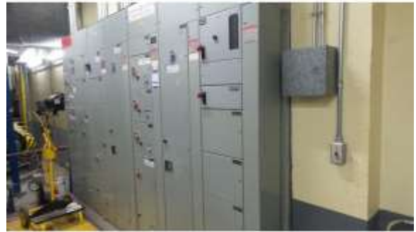
BROD068e 4/19/2016 600 amp motor control center MCC-BE Room GW58
