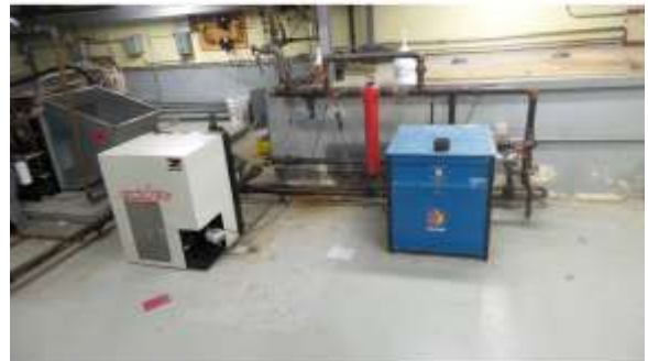
BROD057e 4/19/2016 Air dryers Room GW58
