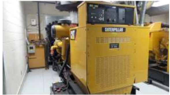
BROD093e 4/19/2016 625 kVA emergency generator #1 Generator building
