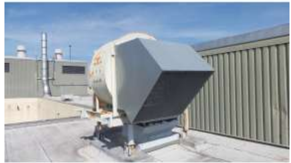
BROD003e 4/19/2016 Utility-set smoke exhaust fan P9 Upper roof
