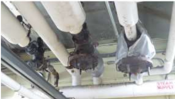
BROD080e 4/19/2016 Pressure reducing valves Room GW58
