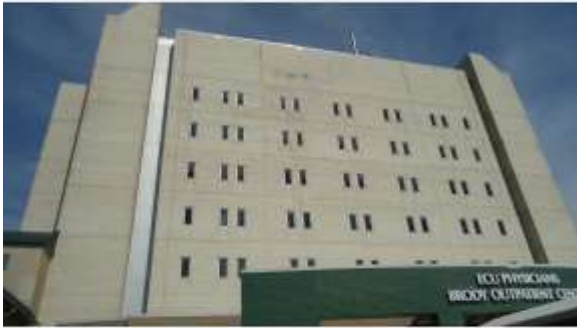
BROD067a 4/19/2016 Exterior masonry has moisture penetration issues Exterior
