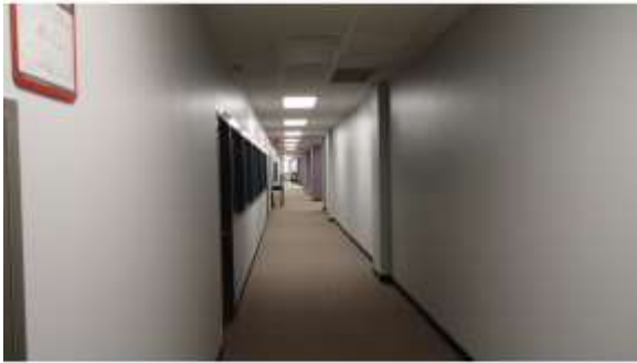
BROD047a 4/19/2016 Carpeted corridor with painted walls and suspended grid ceilings Second floor
