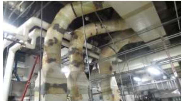
BROD032e 4/19/2016 Duct work exposed to perchloric acid fumes Room 8N08
