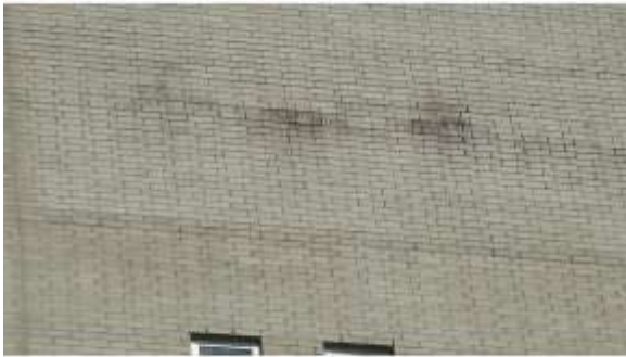
BROD068a 4/19/2016 Exterior masonry has moisture penetration issues Exterior
