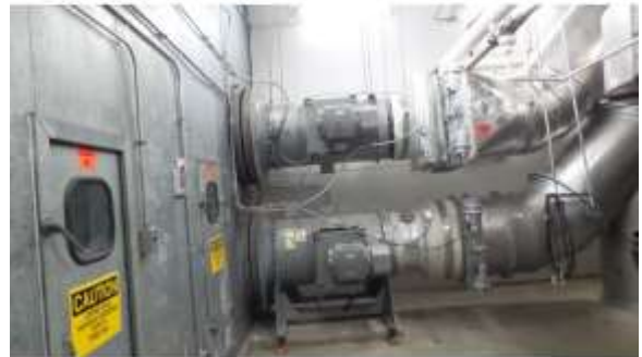
BROD023e 4/19/2016 Updated inline fans 8-68 and 8-69 Room 8N08
