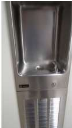
BROD030a 4/19/2016 Built-in single-level water fountain Seventh floor
