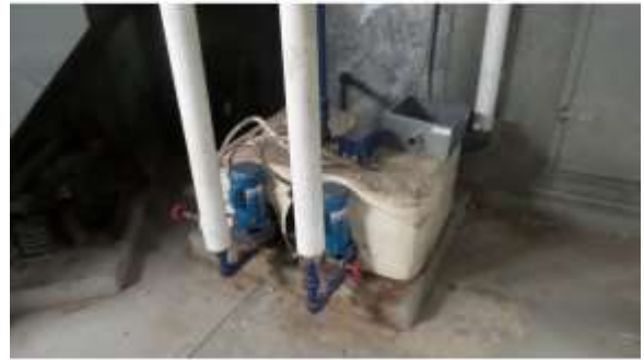
BROD065e 4/19/2016 AHU AC2 condensate return unit Room GW58
