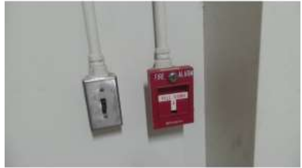
BROD016e 4/19/2016 Fire alarm system pull station Room 8N08
