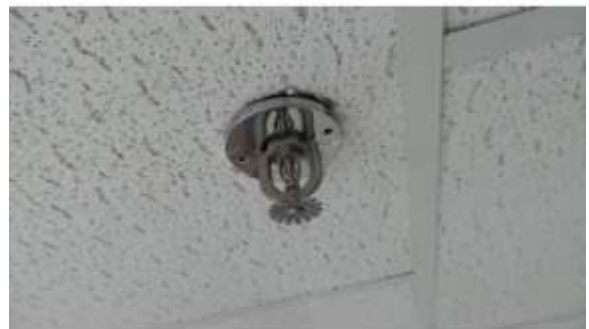
BROD048e 4/19/2016 Original fire system sprinkler head Eighth floor, corridor
