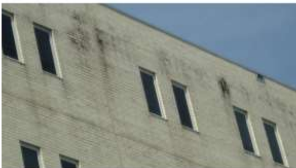
BROD072a 4/19/2016 Exterior masonry has moisture penetration issues Exterior
