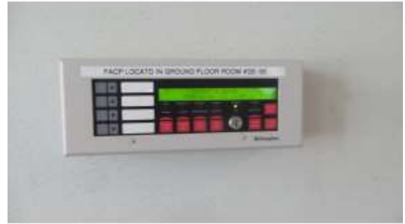
BROD103e 4/19/2016 Fire alarm system annunciator panel First floor, main entry
