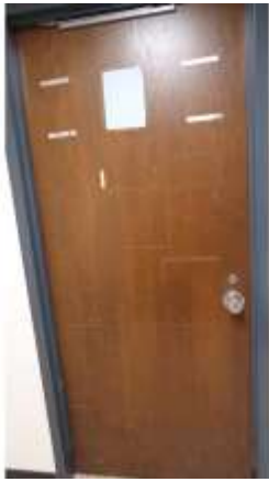
BROD043a 4/19/2016 Knob actuated door hardware and no signage Fifth floor
