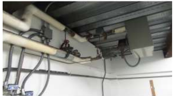
BROD009e 4/19/2016 Original hydronic unit heater South elevator machine room
