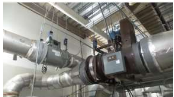
BROD018e 4/19/2016 Inline fans Room 8N08
