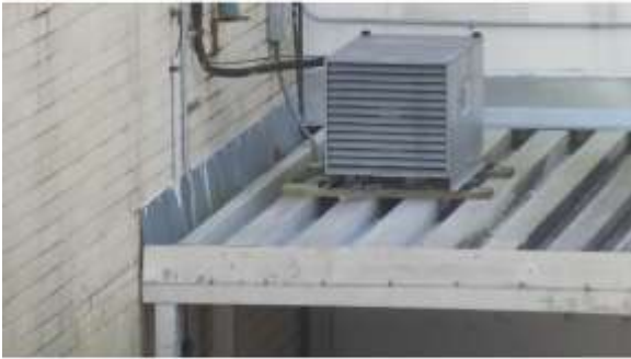
BROD102e 4/19/2016 Walk-in cooler refrigeration equipment Exterior
