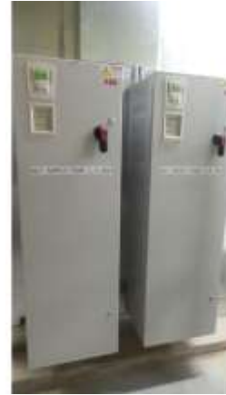
BROD071e 4/19/2016 AHU AC1 supply fan wall VFD's Room GW58
