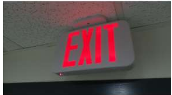
BROD051e 4/19/2016 Updated exit signage with LED lamp Eighth floor, corridor
