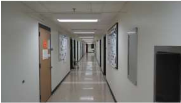
BROD029a 4/19/2016 Vinyl tile in corridors, with suspended grid ceilings and painted walls Seventh floor
