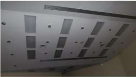
BROD104e 4/19/2016 Original auditorium lighting system Auditorium
