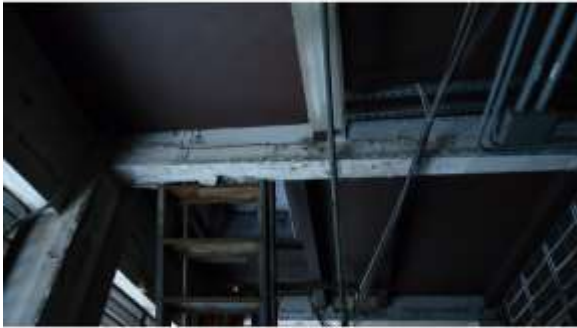
BROD013a 4/19/2016 Poor coating on steel superstructure Penthouse
