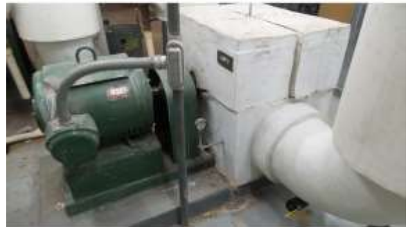
BROD074e 4/19/2016 75 hp chilled water pump Room GW58
