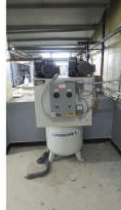
BROD056e 4/19/2016 Duplex vacuum pump system Room GW58
