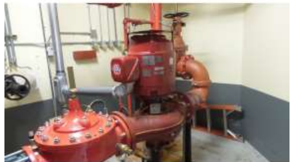
BROD072e 4/19/2016 60 hp fire pump Ground floor, fire pump room
