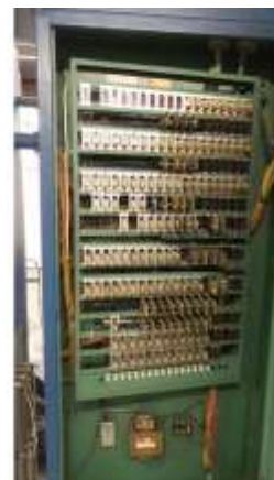
BROD012e 4/19/2016 Passenger elevator control cabinet South elevator machine room
