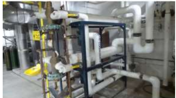
BROD036e 4/19/2016 Domestic water system heat exchanger Room 8S09
