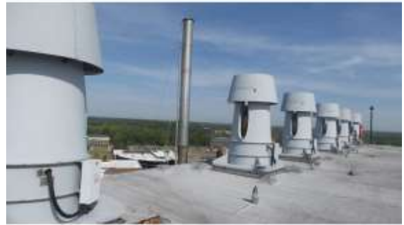
BROD014e 4/19/2016 Updated strobic air fan systems Upper roof
