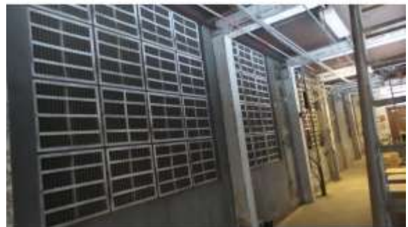
BROD015e 4/19/2016 Filter racks for air handlers Penthouse, mechanical room
