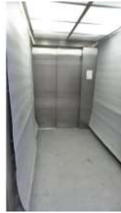
BROD049e 4/19/2016 South freight elevator car Room 8S07
