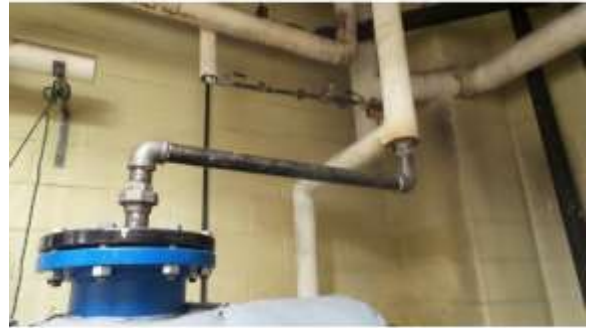
BROD077e 4/19/2016 Improper pipe bend at vacuum condensate system Room GW58
