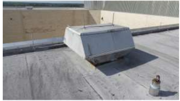
BROD001e 4/19/2016 Roof ventilator Upper roof
