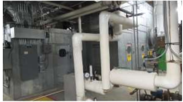
BROD022e 4/19/2016 Air handler AC7 Room 8N08
