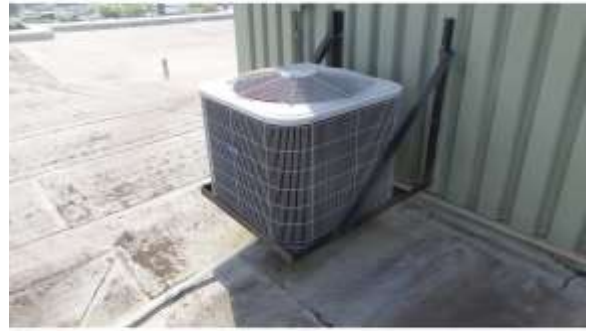
BROD002e 4/19/2016 Air-cooled condenser Upper roof
