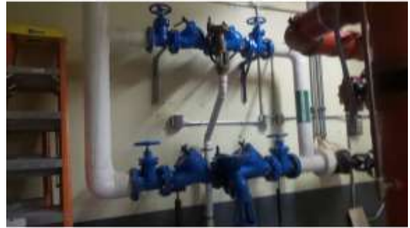
BROD073e 4/19/2016 Domestic water backflow preventers Ground floor, fire pump room
