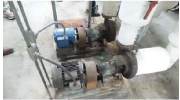
BROD025e 4/19/2016 Original pumps Room 8N08
