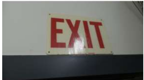
BROD042e 4/19/2016 Radioluminescent tritium exit signage Room 8S08B
