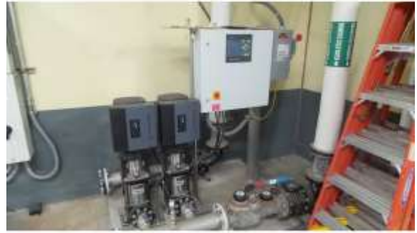
BROD070e 4/19/2016 Domestic water booster pump system Room GW58
