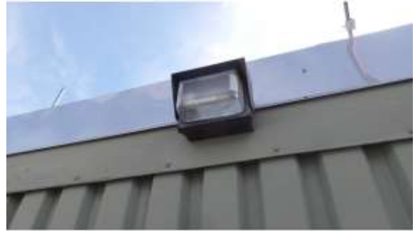
BROD013e 4/19/2016 Wall-mounted exterior light with HID lamp Upper roof
