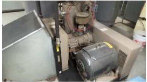
BROD067e 4/19/2016 Air compressor Room GW58
