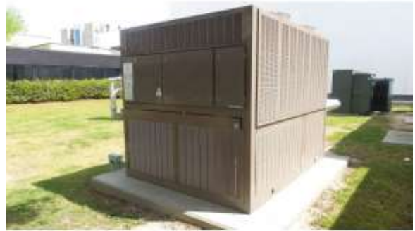
BROD091e 4/19/2016 Air-cooled chiller Exterior
