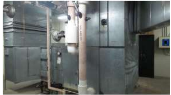
BROD087e 4/19/2016 Air handler 88-2 Room 3E144
