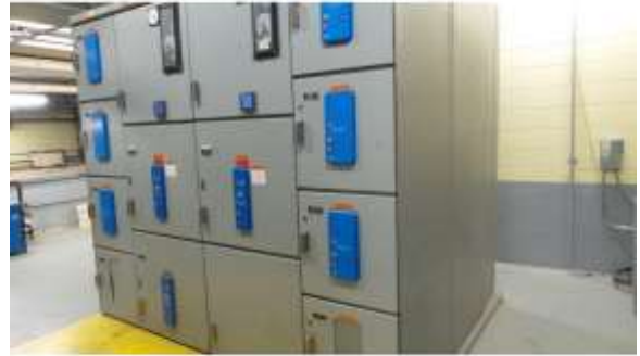
BROD061e 4/19/2016 3,200 amp substation SSB Room GW58
