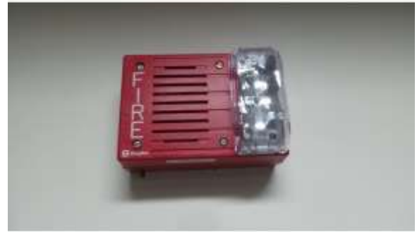
BROD050e 4/19/2016 Fire alarm system visual and audible device Eighth floor, corridor
