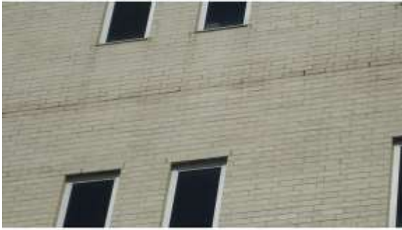
BROD070a 4/19/2016 Exterior masonry has moisture penetration issues Exterior
