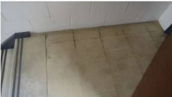
BROD033a 4/19/2016 Aged floor tile Stairwell landing
