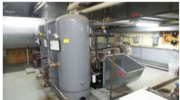
BROD066e 4/19/2016 Compressed air storage tanks Room GW58
