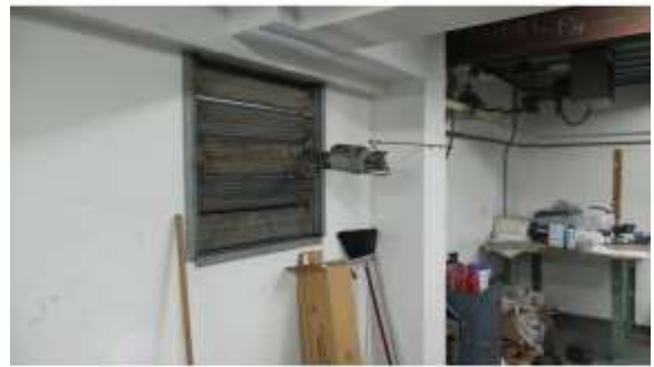
BROD008e 4/19/2016 Pneumatic damper South elevator machine room
