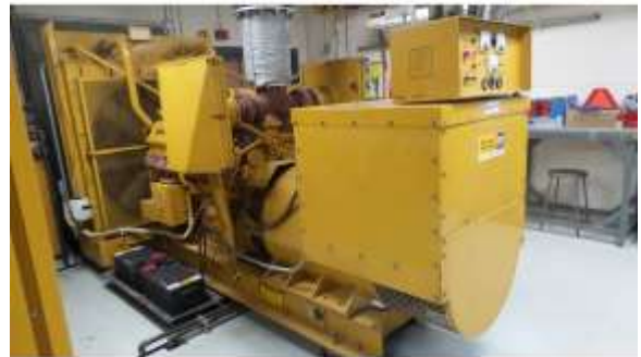
BROD095e 4/19/2016 600 kW emergency generator #3 Generator building
