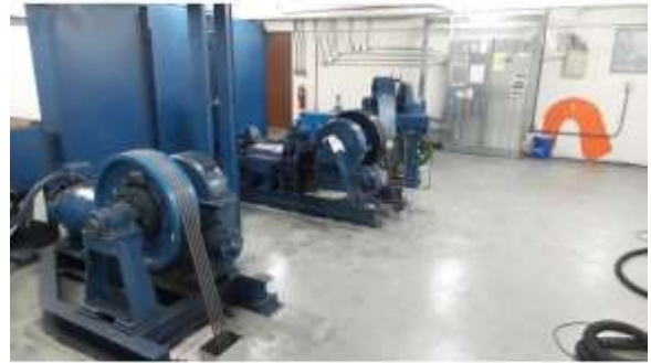
BROD005e 4/19/2016 Original traction elevator machines South elevator machine room
