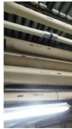
BROD058e 4/19/2016 Miscellaneous distribution piping Room GW58
