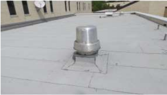
BROD090e 4/19/2016 Centrifugal rooftop exhaust fans Lower roof
