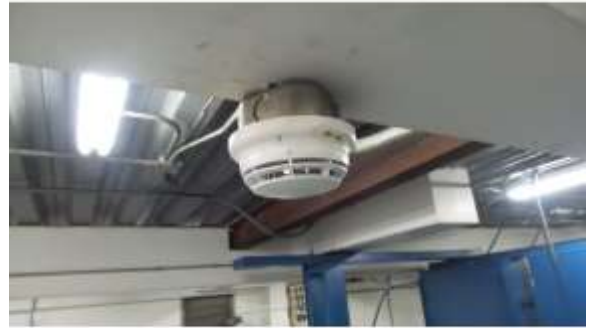
BROD007e 4/19/2016 Updated smoke/heat detector South elevator machine room
