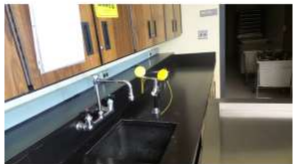
BROD054e 4/19/2016 Eyewash/drench hose station Room 8E18
