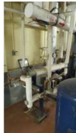
BROD075e 4/19/2016 Instantaneous water heater/heat exchanger Room GW58
