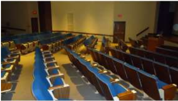
BROD059a 4/19/2016 Terraced auditorium without adequate aisle handrails First floor
