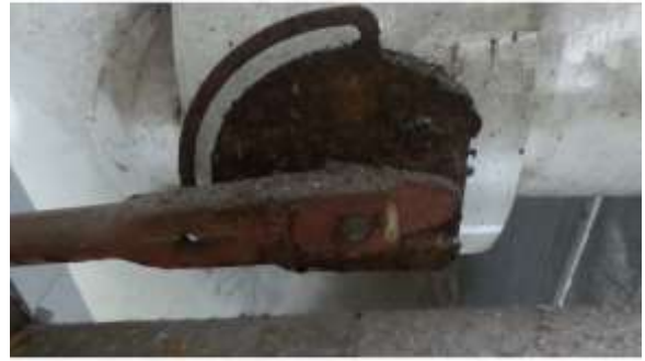
BROD028e 4/19/2016 Moderate corroded chilled water butterfly valve Room 8N08
