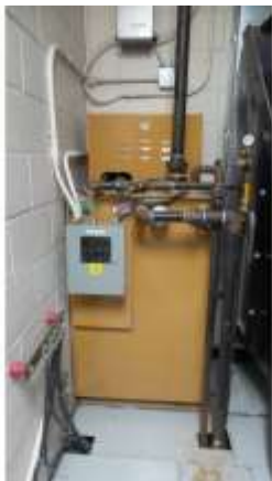
BROD094e 4/19/2016 Fuel oil day tank Generator building
