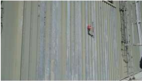
BROD010a 4/19/2016 Poor paint finish on corrugated metal exterior panels Penthouse
