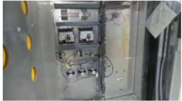
BROD019e 4/19/2016 Air handler AC6 control cabinet Room 8N08
