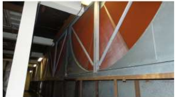
BROD089e 4/19/2016 Energy recovery wheels Penthouse, mechanical room
