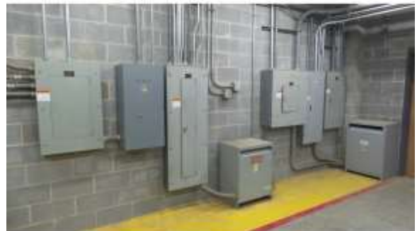
BROD045e 4/19/2016 Miscellaneous secondary electrical equipment Room 8S08B
