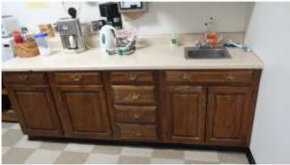
BROD041a 4/19/2016 Aged wooden cabinetry and original stainless sink Fifth floor, break room
