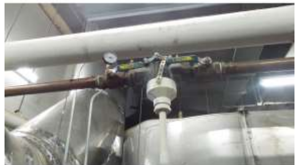
BROD024e 4/19/2016 Cooling return bypass backflow preventer Room 8N08
