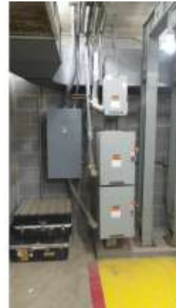
BROD044e 4/19/2016 Original 480/277 volt bus plugs Room 8S08B
