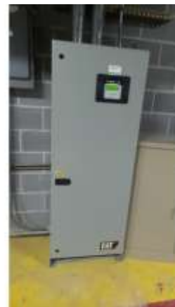
BROD027e 4/19/2016 480/277 volt automatic transfer switch Room 8N08A
