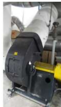
BROD021e 4/19/2016 Utility set fan 8-75 Room 8N08
