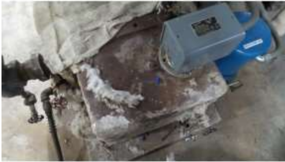
BROD084e 4/19/2016 Damaged insulation on condensate unit Room GL02
