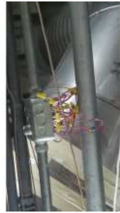
BROD034e 4/19/2016 Exposed secondary electrical wiring Room 8N08
