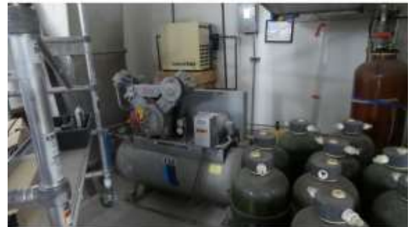
BROD038e 4/19/2016 Original air compressor and updated air dryer Room 8S09
