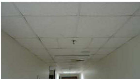
BROD018a 4/19/2016 Aged suspended grid ceiling system Eighth floor
