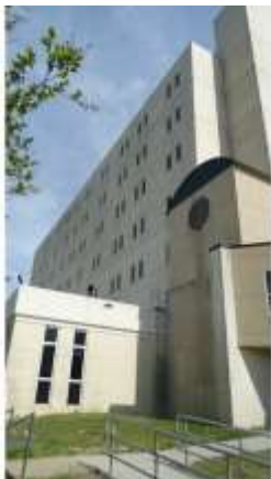
BROD063a 4/19/2016 Exterior staining on the concrete and brick masonry veneer finish Exterior
