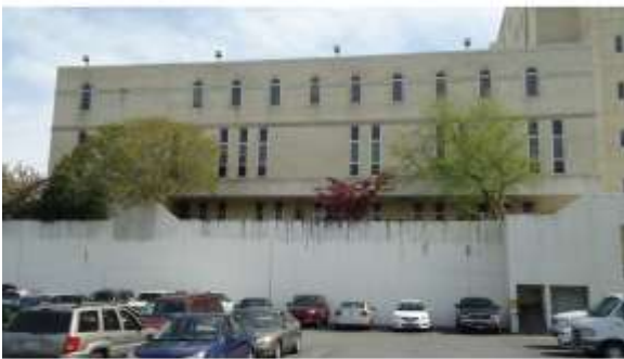
BROD078a 4/19/2016 Exterior staining on the concrete and brick masonry veneer finish Exterior
