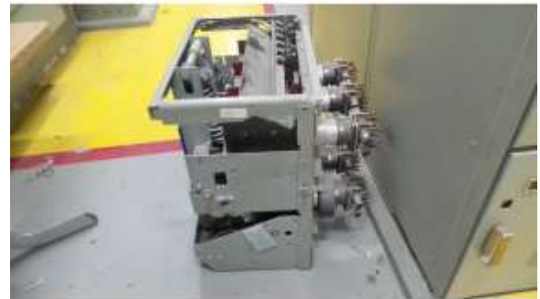
BROD060e 4/19/2016 Original power circuit breaker, spare Room GW58
