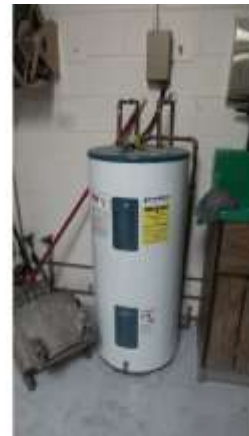
BROD099e 4/19/2016 Electric domestic water heater Generator building
