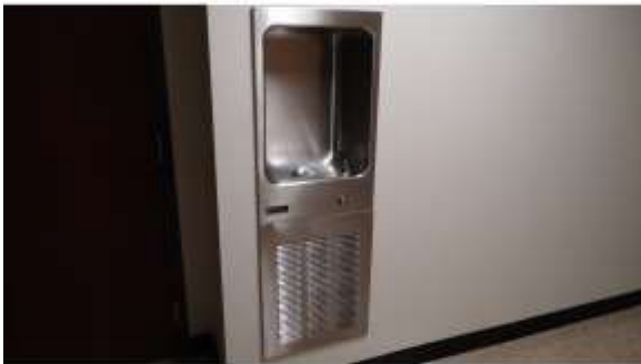
BROD017a 4/19/2016 Built-in single-level drinking fountain Eighth floor
