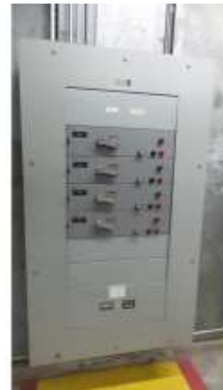
BROD030e 4/19/2016 Motor controller 8SPF Room 8N08
