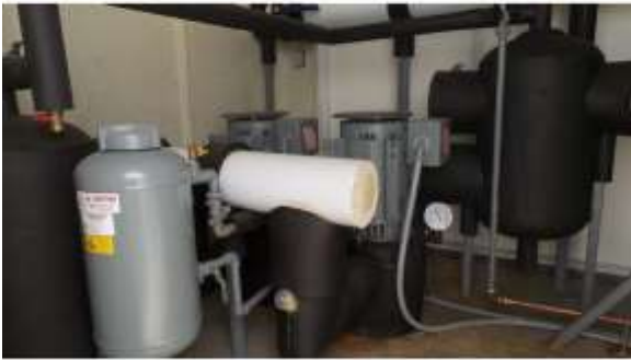
BROD092e 4/19/2016 Chilled water pumps Exterior
