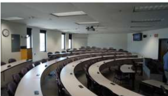
BROD054a 4/19/2016 Terraced classroom without adequate handrails Second floor
