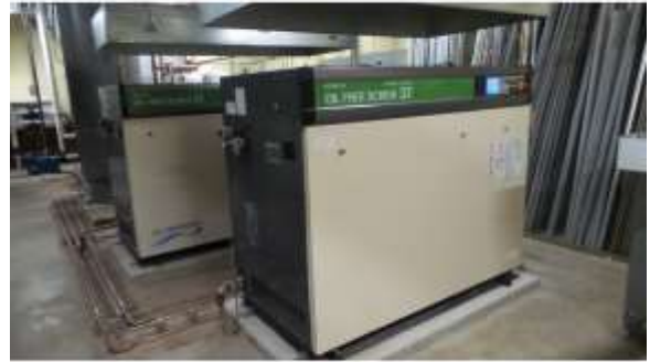
BROD085e 4/19/2016 Screw-type, oil-less air compressors Room GL02
