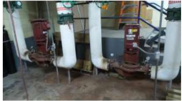
BROD079e 4/19/2016 Heating water pumps 1 and 2 Room GW58
