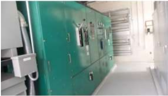
BROD098e 4/19/2016 Original transfer switches Generator building
