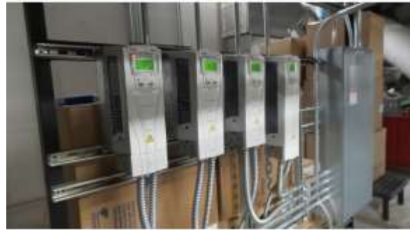
BROD020e 4/19/2016 Miscellaneous variable speed drives Room 8N08
