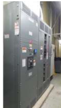
BROD063e 4/19/2016 Updated Square D switchgear SSEB Room GW58
