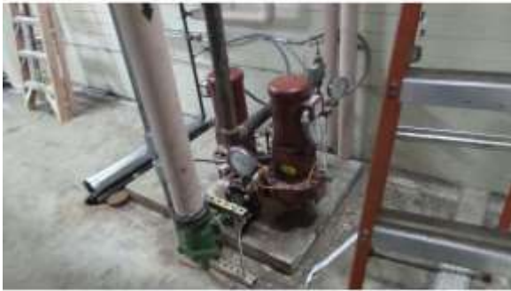
BROD086e 4/19/2016 Heating water pumps Room 3E144
