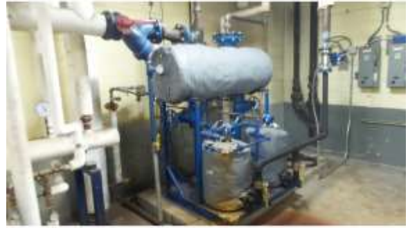
BROD076e 4/19/2016 Vacuum condensate return system Room GW58
