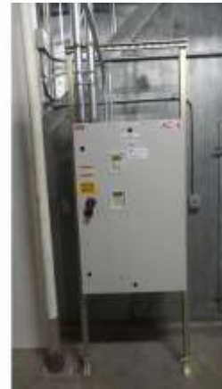
BROD017e 4/19/2016 Variable speed drive air handler supply AC6 Room 8N08
