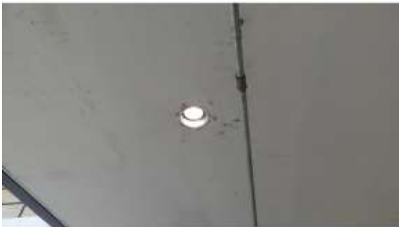
BROD100e 4/19/2016 Recessed exterior light fixture Loading dock
