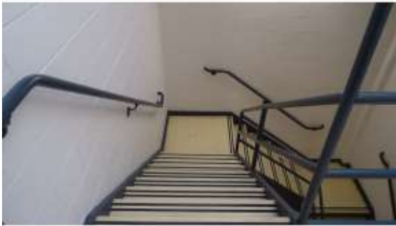
BROD014a 4/19/2016 Compliant handrails without adequate guardrail protection Stairwell
