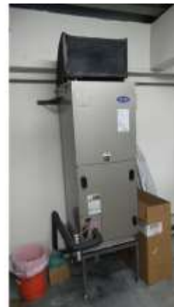
BROD010e 4/19/2016 Air handler South elevator machine room
