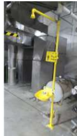
BROD035e 4/19/2016 Emergency shower/eyewash station Room 8S09
