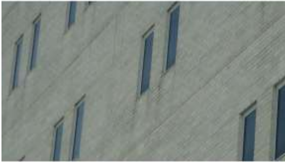
BROD064a 4/19/2016 Exterior staining on the brick masonry veneer finish Exterior
