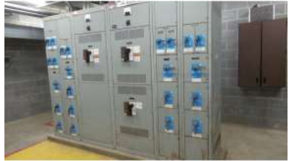
BROD043e 4/19/2016 Original 1,200 amp main breakers A, B, tie, and switchgear Room 8S08B
