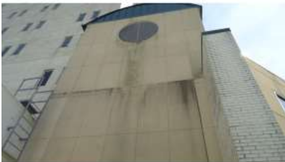
BROD066a 4/19/2016 Exterior staining on the concrete veneer finish Exterior
