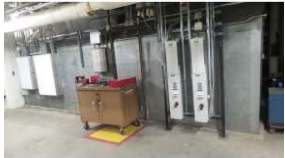
BROD033e 4/19/2016 Air handler AC4, VFDs, and control cabinets Room 8N08
