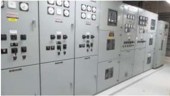
BROD096e 4/19/2016 Emergency power switchgear Generator building
