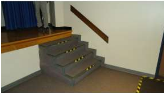
BROD060a 4/19/2016 Steps leading to stage with no handrails First floor
