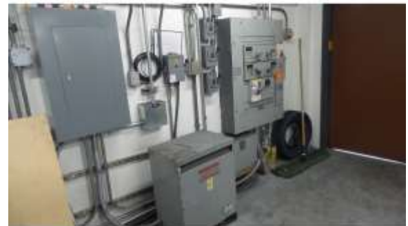
BROD011e 4/19/2016 Updated and original secondary electric equipment South elevator machine room
