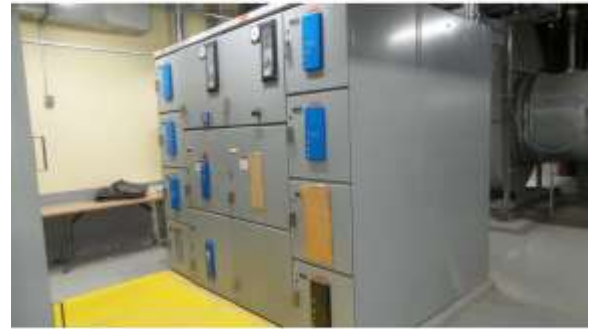
BROD059e 4/19/2016 3,200 amp substation SSA Room GW58
