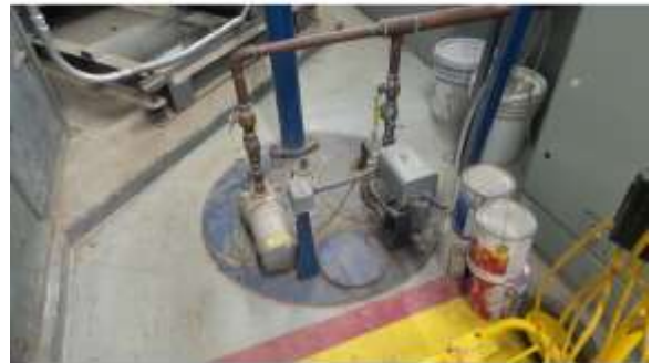
BROD069e 4/19/2016 Submersible sump pumps Room GW58
