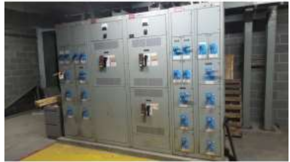
BROD026e 4/19/2016 Original 1,200 amp main breakers C, D, tie, and switchgear Room 8N08A
