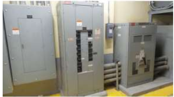
BROD062e 4/19/2016 Secondary electrical equipment Room GW58
