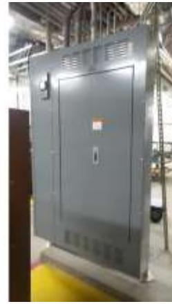
BROD037e 4/19/2016 Updated Square D panelboard Room 8S09
