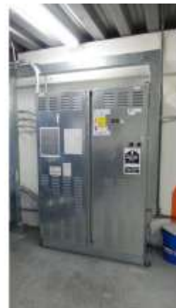
BROD006e 4/19/2016 Updated freight elevator controls South elevator machine room
