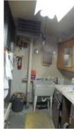
BROD041e 4/19/2016 Utility sink and hydronic heater Room 8S08D
