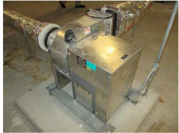
CARD013e 11/6/2018 1/2 hp Loren Cook exhaust fan EF-6 East mezzanine
