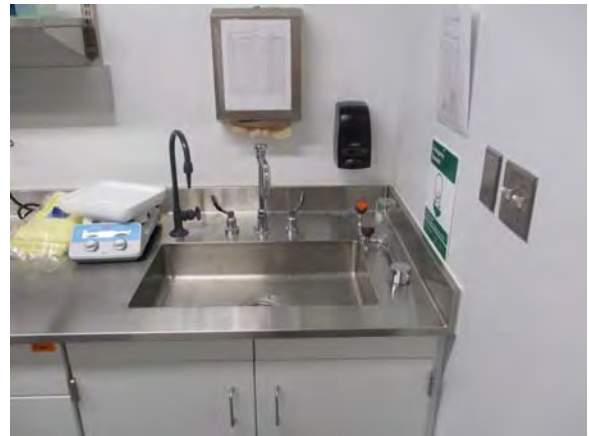
CARD057e 11/6/2018 Eyewash station next to vivarium sink Room 4313F
