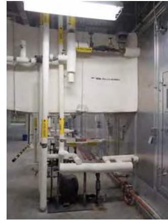
CARD022e 11/6/2018 Steam piping going into the humidification section of AHU-4 Center mezzanine
