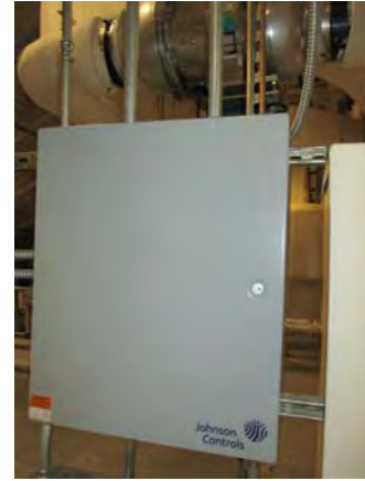
CARD011e 11/6/2018 Enclosure for Johnson Controls HVAC controls East mezzanine
