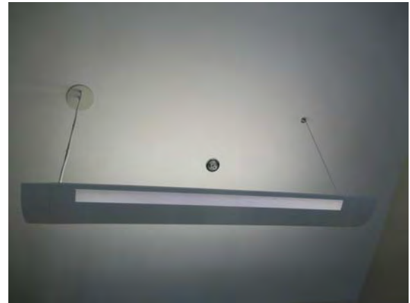
CARD038e 11/6/2018 Pendent fluorescent light fixture and sprinkler head East stairwell
