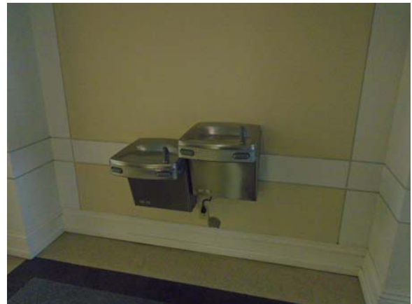
CARD145a 11/6/2018 Dual-level water fountains Corridor 1421
