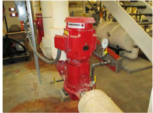
CARD088e 11/6/2018 25 hp heating hot water pump P2-1 Room 1418
