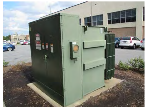
CARD102e 11/6/2018 2,000 kVA oil-filled transformer TX-19 East exterior
