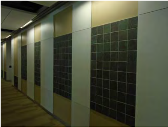
CARD058a 11/6/2018 Carpeting, painted and tiled walls, and suspended ceiling Fourth floor
