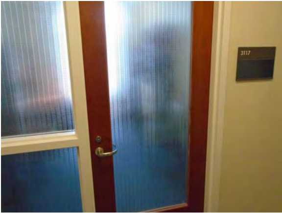
CARD062a 11/6/2018 Glazed interior door with lever hardware and accessible signage Third floor
