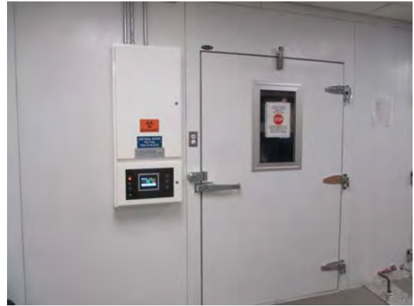
CARD052e 11/6/2018 Walk-in cold room Room 4210B
