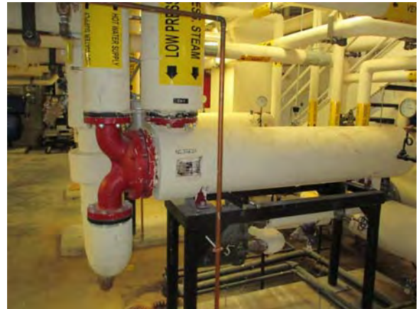
CARD086e 11/6/2018 CV-1 heat exchanger producing heating hot water Room 1418
