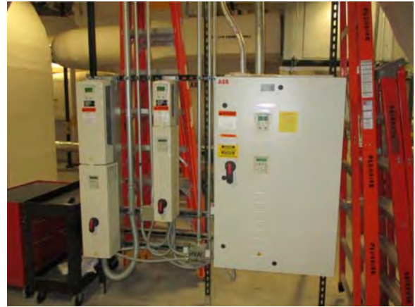
CARD010e 11/6/2018 Group of three ABB variable frequency drives East mezzanine
