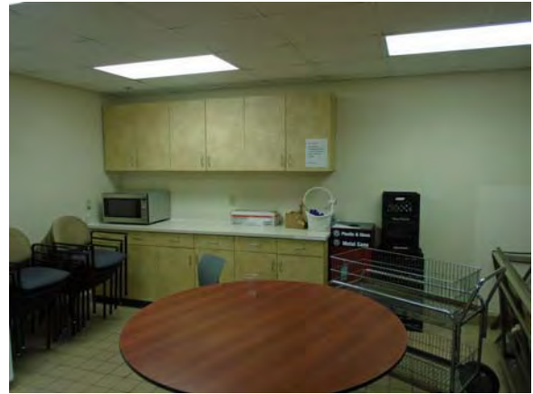
CARD143a 11/6/2018 Tiled floor, painted walls, suspended ceiling, and base and overhead cabinetry Kitchen 1414
