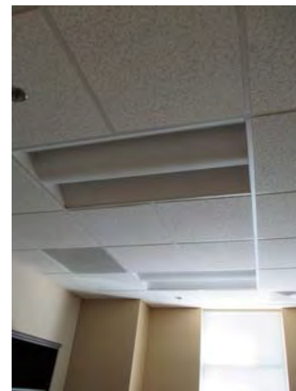
CARD063e 11/6/2018 Lay-in fluorescent light fixtures Office 3121
