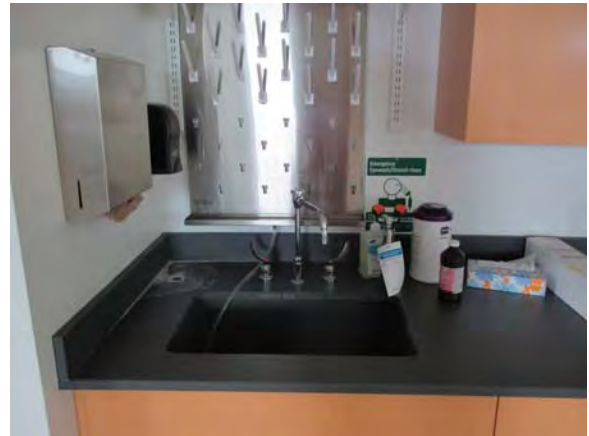
CARD050e 11/6/2018 Emergency eyewash station next to the lab sink Fourth floor surgery room
