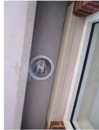
CARD100e 11/6/2018 Ceiling recessed CFL exterior light West exterior
