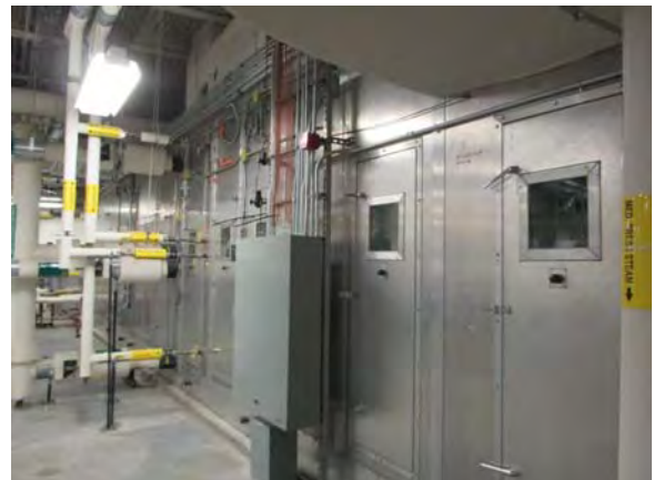
CARD021e 11/6/2018 Large Buffalo air handling unit AHU-4 Center mezzanine
