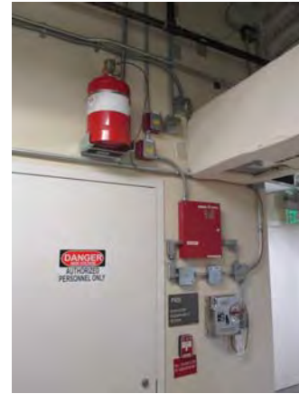
CARD028e 11/6/2018 Dry chemical fire suppression system for elevator equipment room P105 Northwest mezzanine
