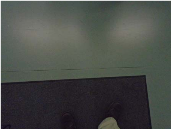
CARD022a 11/6/2018 Seams opening up in sheet flooring Fourth floor
