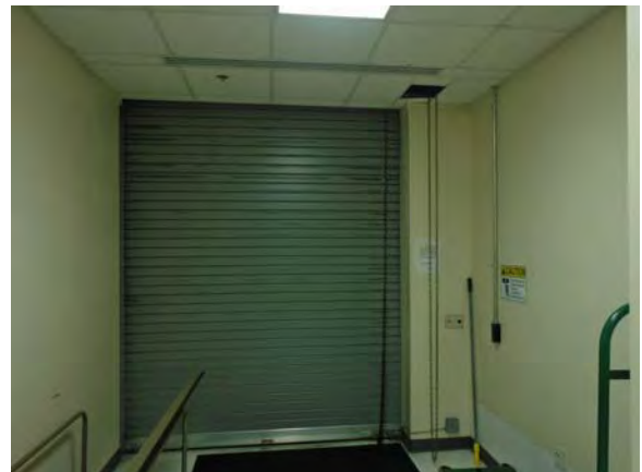
CARD153a 11/6/2018 Overhead roll-up service door Shipping/receiving 1419
