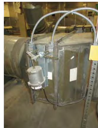
CARD024e 11/6/2018 Pneumatic actuator on EF-1-2 Center mezzanine
