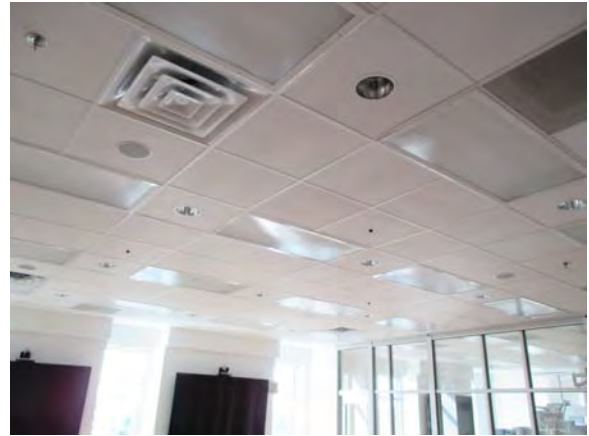
CARD049e 11/6/2018 Modern lay-in fluorescent light fixtures Conference room 4200
