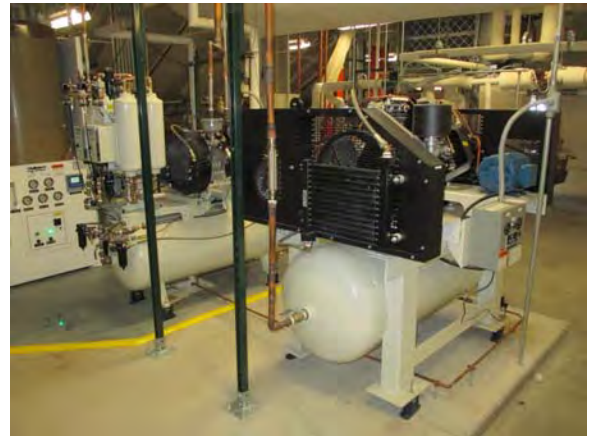
CARD035e 11/6/2018 Powerex air compressor systems AC1 and AC2 East mezzanine
