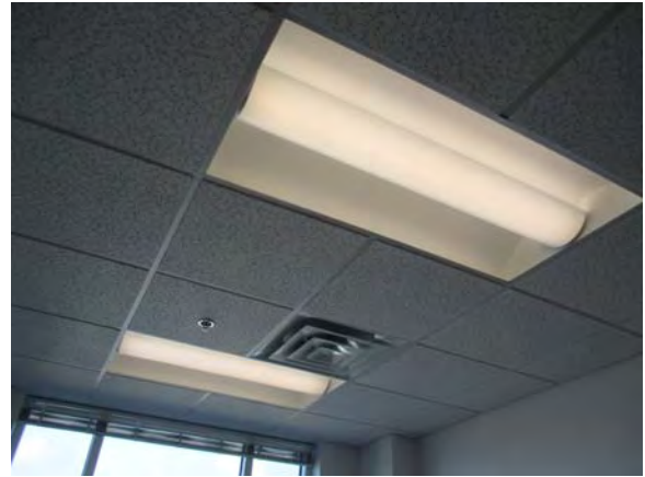
CARD061e 11/6/2018 Modern lay-in fluorescent light fixtures Office 4106
