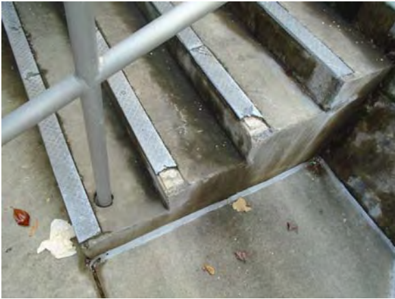
CARD184a 11/6/2018 Broken nosing on exterior steps Southeast exterior
