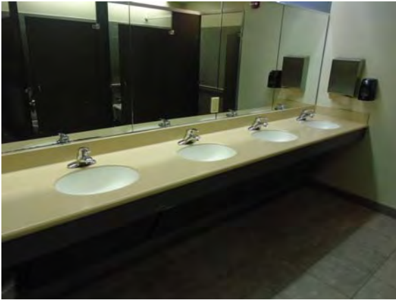
CARD136a 11/6/2018 Tiled floor and walls and accessible lavatories First floor men's restroom
