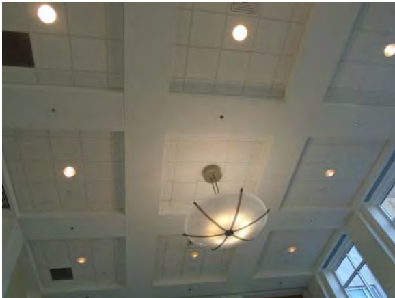
CARD156a 11/6/2018 Suspended grid ceiling system Prefunction space 1408
