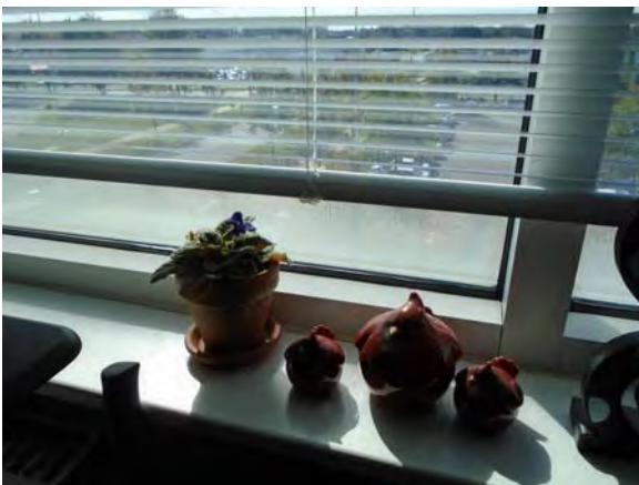
CARD063a 11/6/2018 Condensation collecting between glass panes with lost seal Third floor
