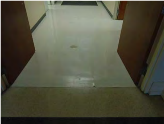
CARD160a 11/6/2018 Interface between terrazzo and sheet vinyl flooring Corridor 1420
