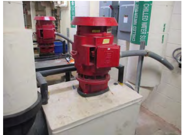
CARD077e 11/6/2018 Two 40 hp chilled water pumps Room 1418
