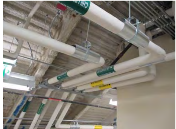
CARD002e 11/6/2018 Insulated piping (chilled and heating hot water) Northeast mezzanine
