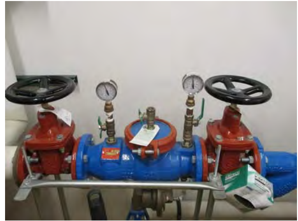
CARD046e 11/6/2018 2 inch domestic water backflow preventer Room 4005
