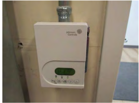
CARD041e 11/6/2018 Johnson Controls digital thermostat Room 4004
