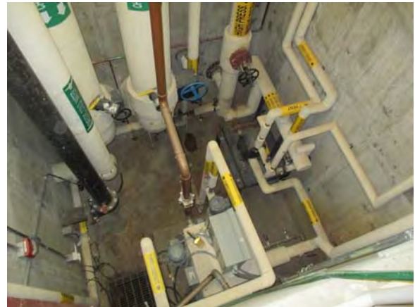
CARD080e 11/6/2018 Pit for chilled water and steam/condensate piping Room 1418
