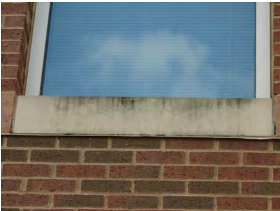
CARD180a 11/6/2018 Concrete windowsills with superficial cracking Southeast exterior
