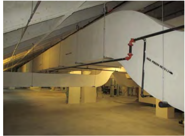
CARD014e 11/6/2018 HVAC ductwork South mezzanine
