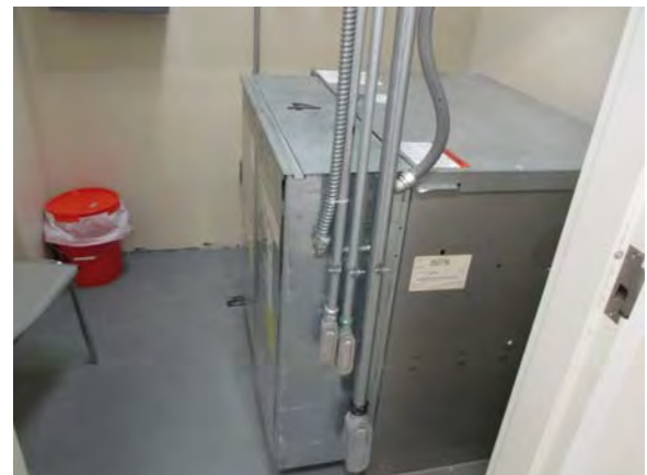
CARD030e 11/6/2018 50 hp Otis hydraulic pump for elevator 4 P105
