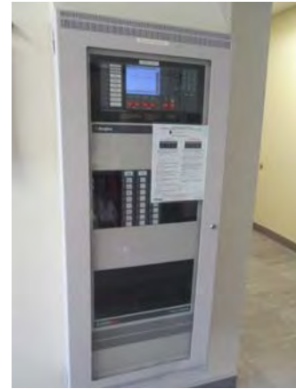
CARD070e 11/6/2018 Simple 4100U fire alarm control panel Vestibule at east entrance
