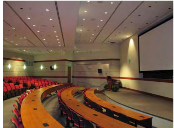
CARD073e 11/6/2018 Recessed can light fixtures Auditorium
