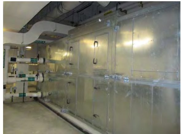
CARD015e 11/6/2018 ERU-1 manufactured by Air Zone International South mezzanine
