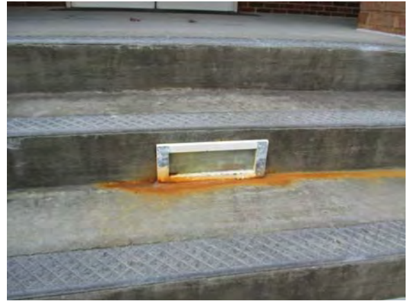
CARD104e 11/6/2018 Corroding exterior step light East exterior
