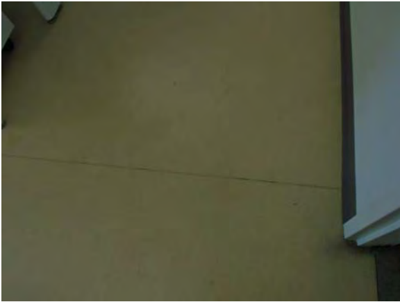
CARD041a 11/6/2018 Seams opening up in sheet flooring Fourth floor
