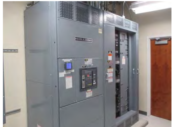
CARD069e 11/6/2018 3,000 amp, 480 V Square D main distribution panel Room 1118
