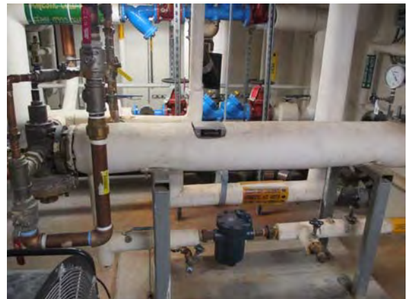
CARD078e 11/6/2018 ThermaFlo domestic water heat exchanger Room 1418
