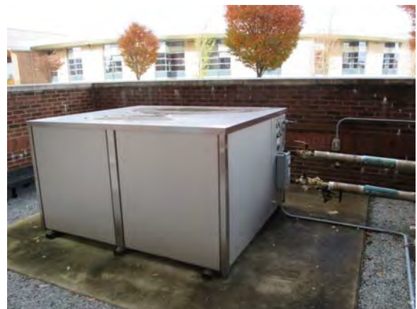
CARD099e 11/6/2018 Chiller for CT scan equipment West exterior
