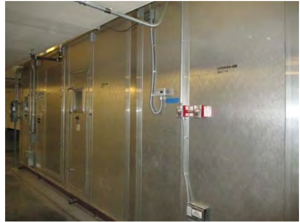
CARD019e 11/6/2018 Return air fan for Buffalo air handling unit AHU-4 Center mezzanine
