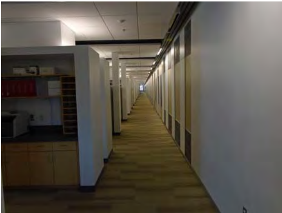
CARD053a 11/6/2018 Carpeting, painted and tiled walls, and suspended ceiling Fourth floor
