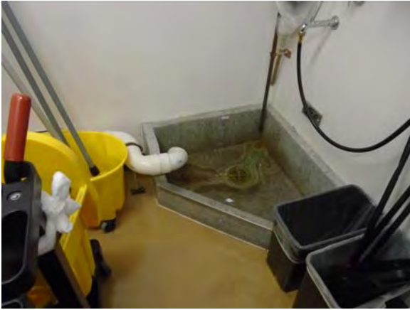
CARD011a 11/6/2018 Custodial floor sink Fourth floor
