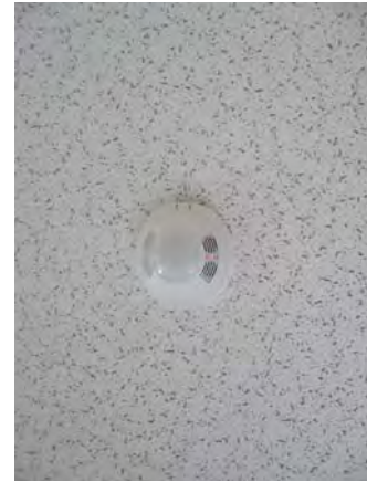
CARD043e 11/6/2018 Modern occupancy sensor Fourth floor corridor
