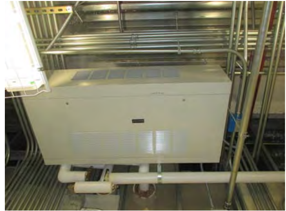
CARD040e 11/6/2018 Fan coil unit cooling the fourth floor electrical room Room 4004
