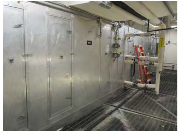
CARD089e 11/6/2018 Air handling unit AHU-1 Room 1418
