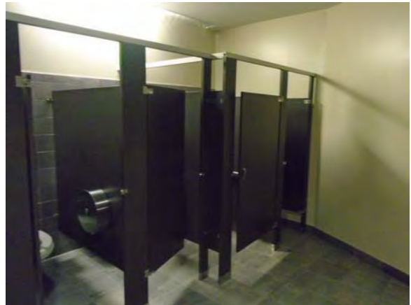
CARD157a 11/6/2018 Tiled floor and walls and accessible water closet stalls Auditorium restroom
