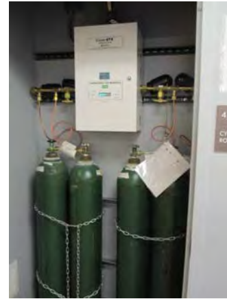
CARD055e 11/6/2018 Cylinder storage with a medical gas control panel Room 4212A
