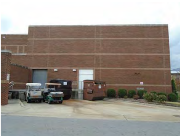
CARD186a 11/6/2018 Brick masonry exterior, overhead service door, and metal personnel doors Southeast exterior
