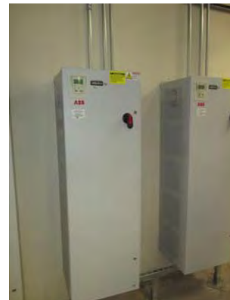
CARD087e 11/6/2018 ABB variable frequency drive for heating hot water P2-1 Room 1418
