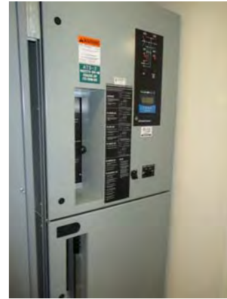
CARD091e 11/6/2018 GE Zenith automatic transfer switch ATS-2 Room 1419E
