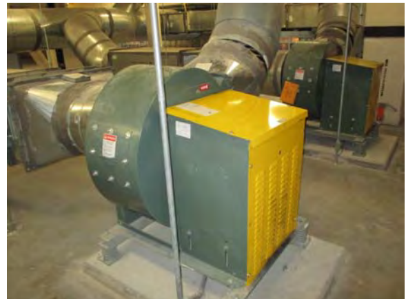
CARD023e 11/6/2018 5 hp exhaust fan EF-1-1 Center mezzanine
