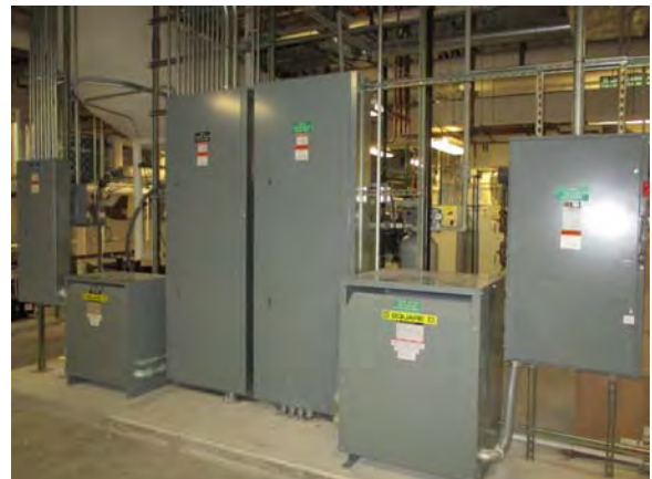
CARD009e 11/6/2018 Square D secondary electrical panels and branch transformers East mezzanine
