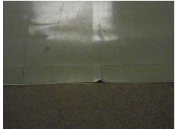
CARD161a 11/6/2018 Interface between terrazzo and sheet vinyl flooring Corridor 1420
