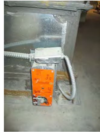
CARD025e 11/6/2018 Electric actuator on the general exhaust ductwork Center mezzanine
