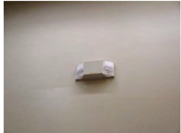
CARD071e 11/6/2018 Unitary emergency light fixture Auditorium conference room
