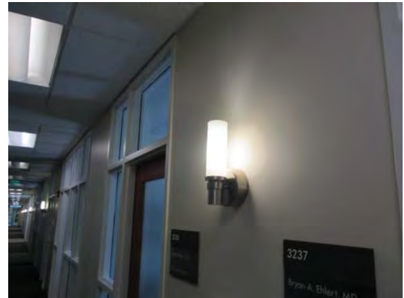
CARD065e 11/6/2018 Wall-mounted sconce light fixture Third floor corridor
