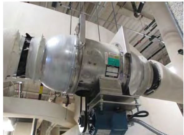
CARD012e 11/6/2018 1.5 hp Loren Cook exhaust fan EF-1 East mezzanine
