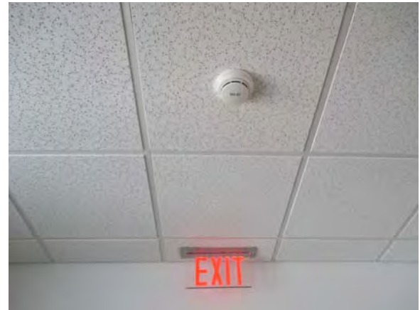
CARD044e 11/6/2018 Modern smoke/heat detector Fourth floor corridor
