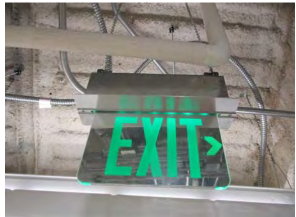
CARD006e 11/6/2018 Edge-lit LED exit sign Northeast mezzanine
