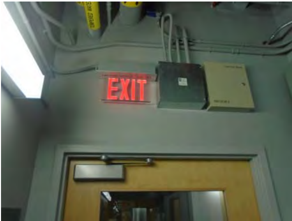
CARD038a 11/6/2018 Illuminated emergency exit signage Fourth floor
