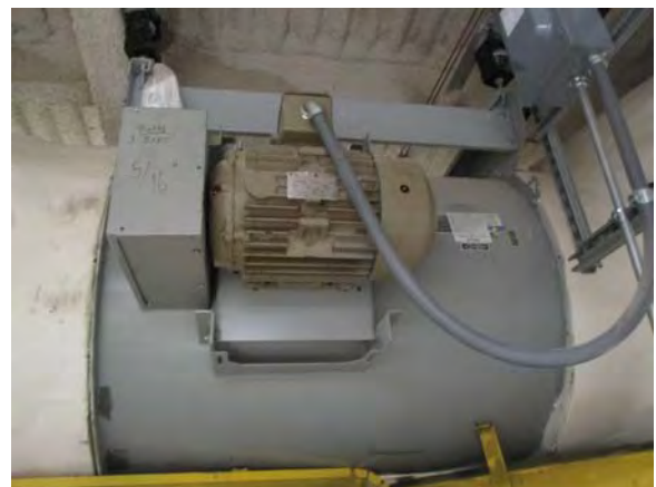
CARD090e 11/6/2018 20 hp return fan for AHU-1 Room 1418
