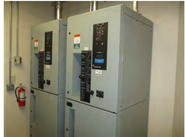
CARD092e 11/6/2018 GE Zenith automatic transfer switches ATS-1A and ATS-1B Room 1419E
