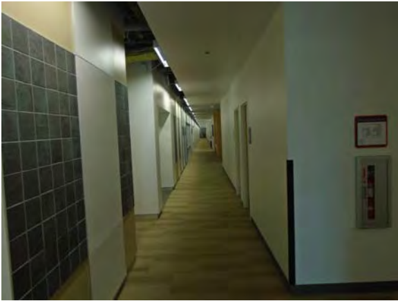
CARD013a 11/6/2018 Carpeting, painted and tiled walls, and painted ceiling (some unfinished areas) Fourth floor corridor
