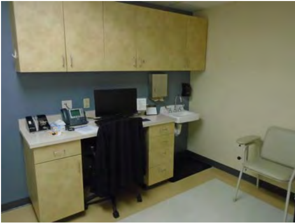
CARD103a 11/6/2018 Vinyl tile floor, painted walls, suspended ceiling, base and overhead cabinetry, and wall-mounted sink Second floor exam room
