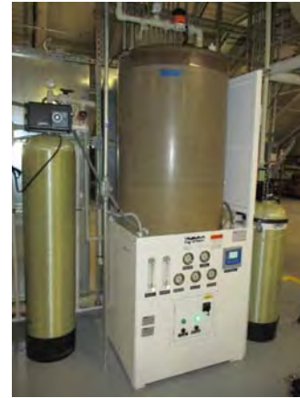
CARD037e 11/6/2018 Hydro RO/DI water treatment system East mezzanine
