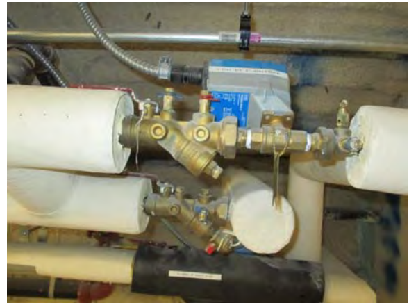
CARD005e 11/6/2018 Electric actuator on the heating hot water return Northeast mezzanine
