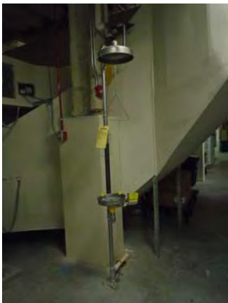
CARD006a 11/6/2018 Emergency eyewash station Penthouse
