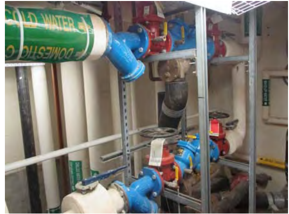
CARD079e 11/6/2018 Two 3 inch backflow preventers for domestic water Room 1418
