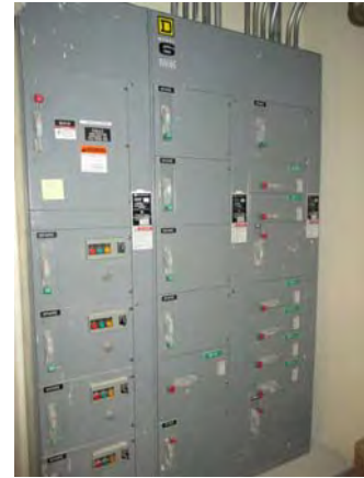
CARD007e 11/6/2018 Square D motor control center Northeast mezzanine
