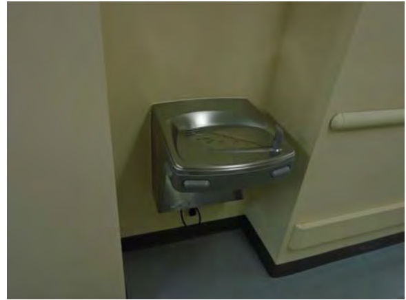
CARD131a 11/6/2018 Single-level water fountain First floor
