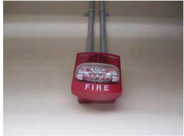
CARD004e 11/6/2018 Modern audible/visible fire alarm device Northeast mezzanine
