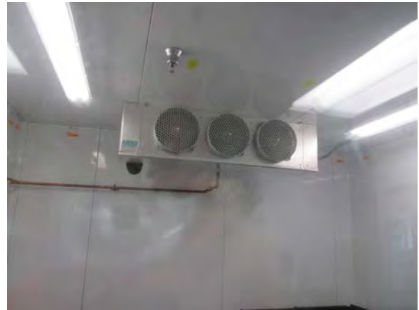
CARD053e 11/6/2018 Three evaporator units inside walk-in cold room Room 4210B
