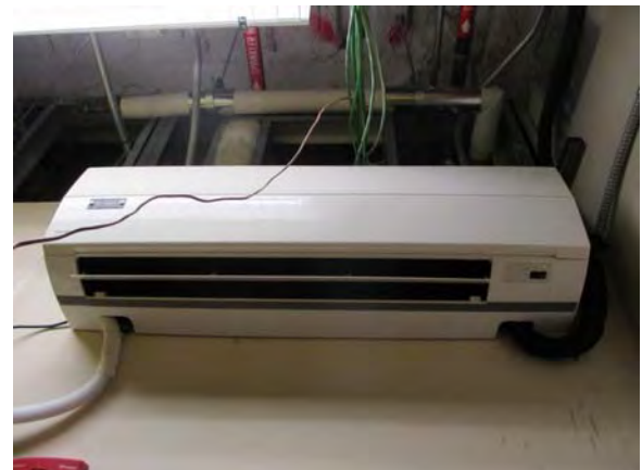
CARD045e 11/6/2018 Evaporator unit for the Toshiba split DX system Room 4003
