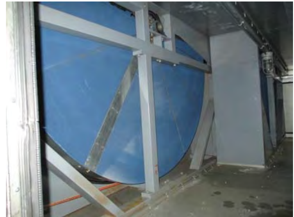
CARD017e 11/6/2018 Energy recovery wheel inside ERU-1 South mezzanine
