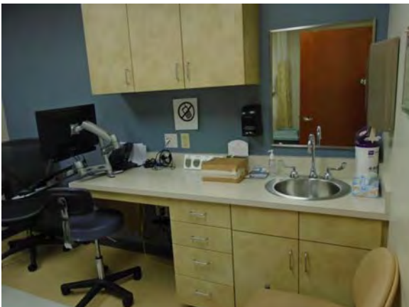
CARD093a 11/6/2018 Vinyl tile floor, painted walls, suspended ceiling, and base and overhead cabinetry with sink Second floor exam room
