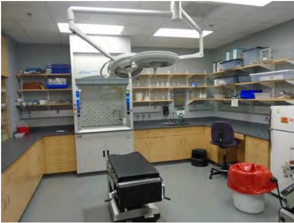
CARD026a 11/6/2018 Sheet vinyl flooring, painted walls, suspended grid ceiling, and wood cabinetry Fourth floor exam room
