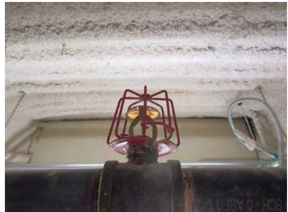
CARD003e 11/6/2018 Sprinkler head Northeast mezzanine
