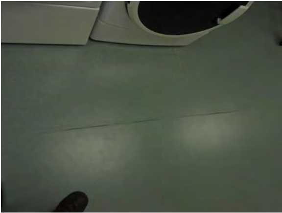
CARD028a 11/6/2018 Seams opening up in sheet flooring Fourth floor
