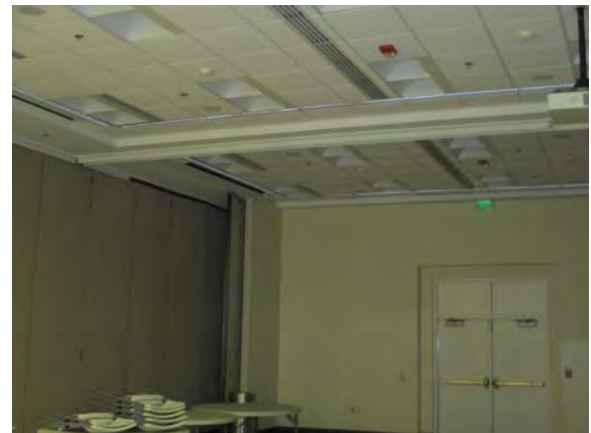
CARD072e 11/6/2018 Lay-in fluorescent light fixtures Auditorium conference room
