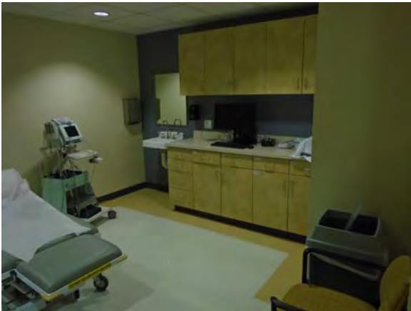
CARD132a 11/6/2018 Vinyl tile floor, painted walls, suspended ceiling, base and overhead cabinetry, and wall-mounted sink First floor exam room
