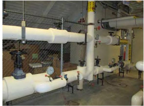
CARD031e 11/6/2018 Pressure reducing valves for the steam piping North mezzanine
