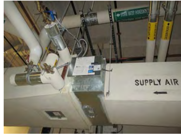
CARD026e 11/6/2018 VAV box and reheat coil inside HVAC ductwork Center mezzanine
