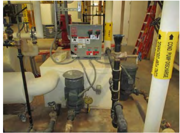
CARD085e 11/6/2018 Condensate pump CP-1 Room 1418
