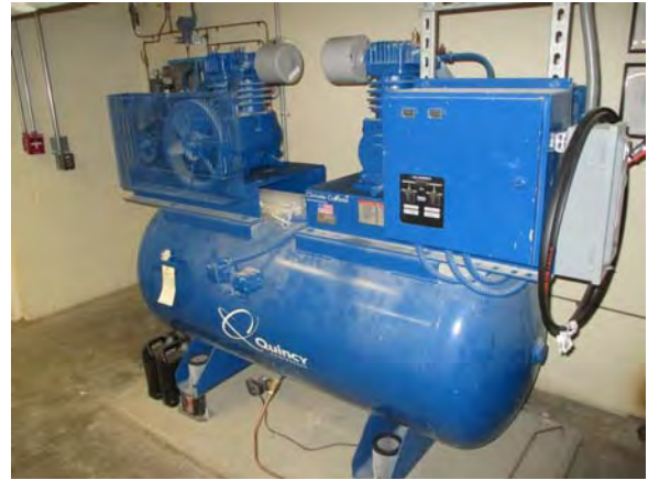
CARD076e 11/6/2018 Quincy air compressor with two 5 hp motors Room 1418
