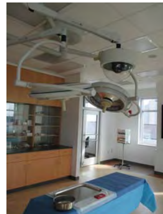
CARD051e 11/6/2018 Special light fixture above surgical table Fourth floor surgery room
