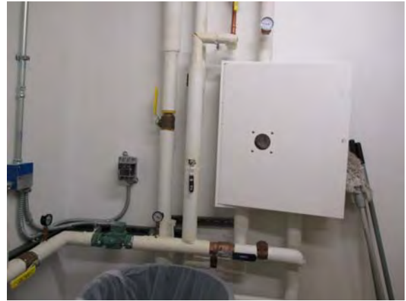
CARD047e 11/6/2018 Mixing valve for the hot/cold water piping Room 4005
