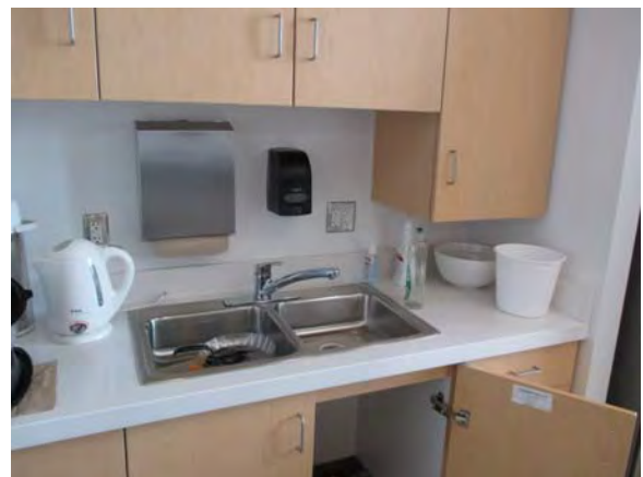
CARD048e 11/6/2018 GFCI protection on electrical outlet near sink Break room 4201
