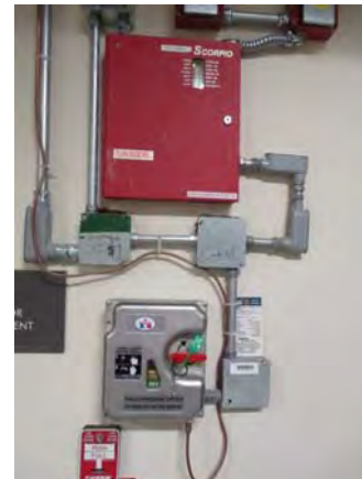
CARD032e 11/6/2018 Kidde control panel for dry chemical fire suppression system for elevator mechanical room P104 Northeast mezzanine
