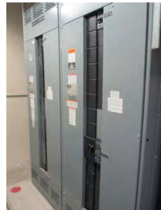
CARD093e 11/6/2018 Square D generator switchboard Room 1419E
