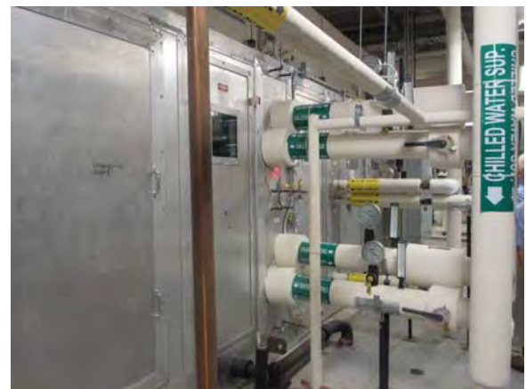
CARD018e 11/6/2018 Large Buffalo air handling unit AHU-2 with incoming water piping (chilled and hot) Center mezzanine
