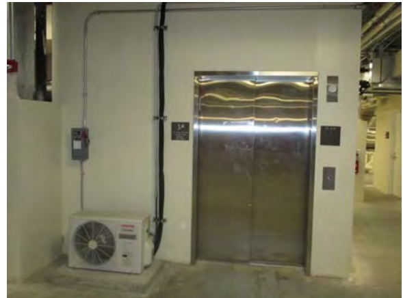
CARD008e 11/6/2018 Toshiba split DX condensing unit adjacent to elevator door Northeast mezzanine
