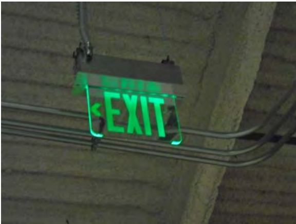
CARD005a 11/6/2018 Illuminated emergency exit sign Penthouse
