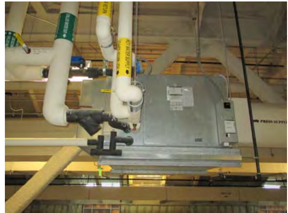
CARD020e 11/6/2018 Fan coil unit P-4 suspended from the ceiling Center mezzanine
