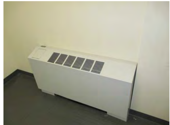
CARD029e 11/6/2018 Fan coil unit S3-P at top of stairwell Northwest stairwell
