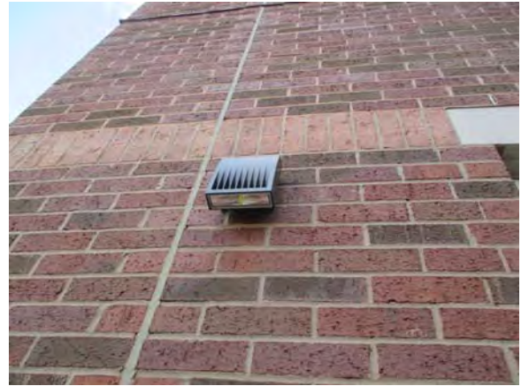
CARD103e 11/6/2018 Wall-mounted LED exterior light East exterior
