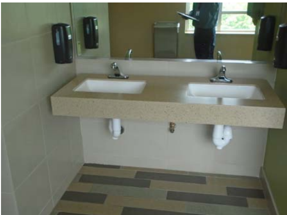
255054a 5/11/2021 Hands-free accessible sinks Restroom
