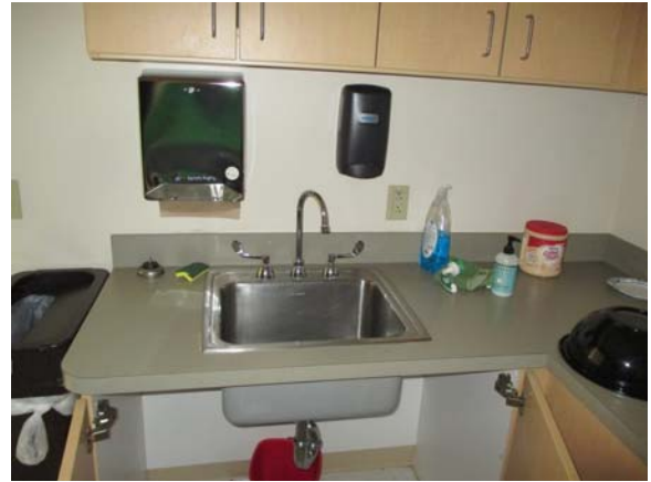
255028e 5/11/2021 Electrical outlet adjacent to sink has GFCI protection Break room 2611C
