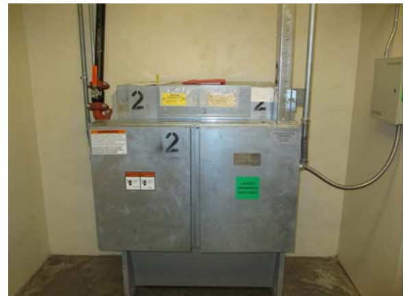
255045e 5/11/2021 Hydraulic pump and controls for one of the Schindler passenger elevators Room L910A
