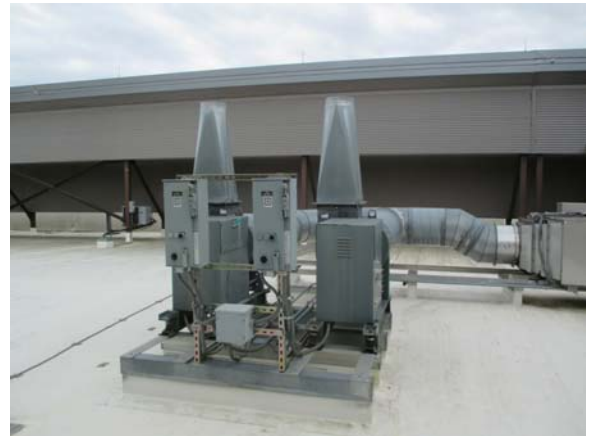
255002e 5/11/2021 5 hp exhaust fans EF-1A and EF-1B Center roof
