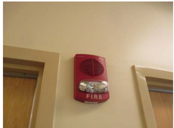
255027e 5/11/2021 Audible/visible fire device Second floor corridor
