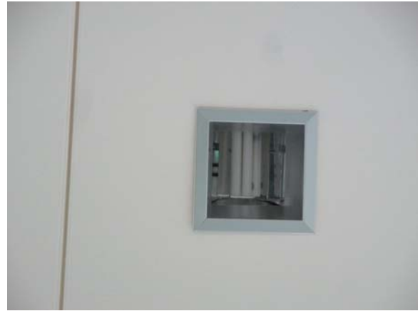
255031e 5/11/2021 Recessed square CFL light fixture Room 2610C
