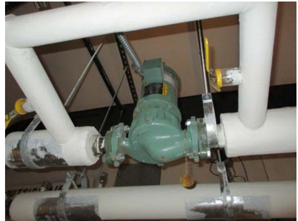
255020e 5/11/2021 Small pump for heating hot water going into AHU-2 Southwest penthouse
