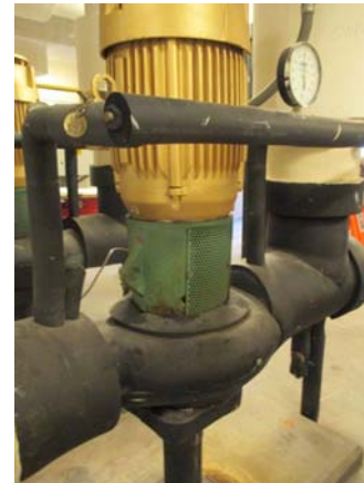
255059e 5/11/2021 25 hp chilled water pump Room L914B
