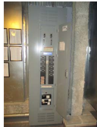
255009e 5/11/2021 Square D secondary electrical panel East penthouse
