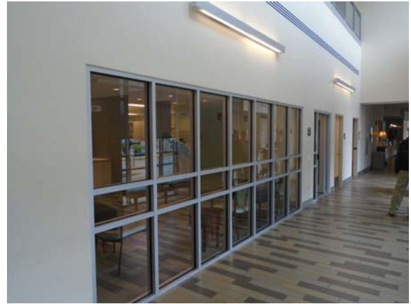
255083a 5/11/2021 Interior partition glazing First floor
