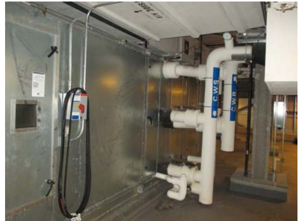
255008e 5/11/2021 Air handling unit AHU-3 with chilled water piping East penthouse
