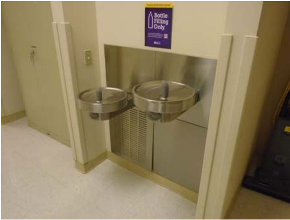
255100a 5/11/2021 Dual-level water fountain First floor
