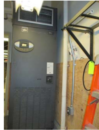
255016e 5/11/2021 Liebert computer room AC unit AHU-9 provides cooling for data/telecom room East penthouse
