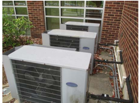
255074e 5/11/2021 Group of three 2.5 ton Carrier condensing units North exterior
