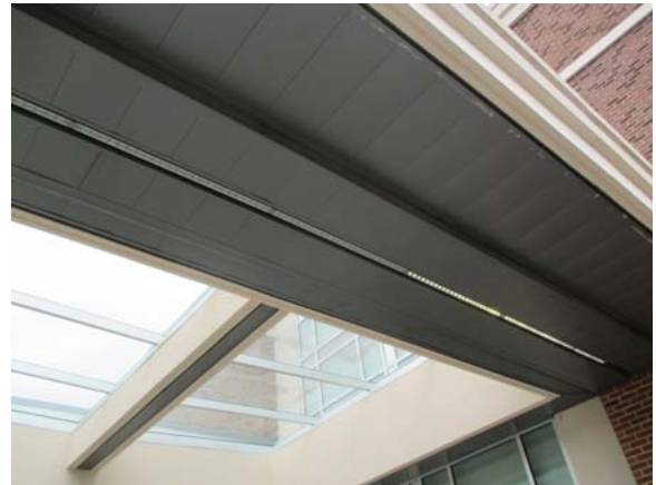
255071e 5/11/2021 Several nonfunctional string LED light fixtures South exterior
