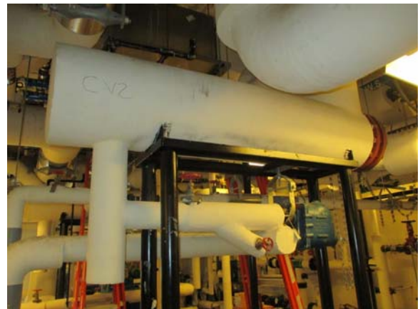
255060e 5/11/2021 CV-2 heat exchanger using steam to produce heating hot water Room L914B
