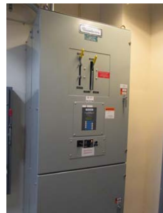
255048e 5/11/2021 Russelectric 600 amp automatic transfer switch ATS-G2 Room L907B
