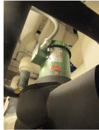
255052e 5/11/2021 2 hp pump CWP-3 Room L914B
