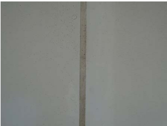
255015a 5/11/2021 Caulked joint with adjacent screws Mechanical penthouse
