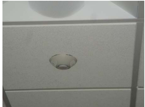
255032e 5/11/2021 Occupancy sensor Large meeting room 2610C
