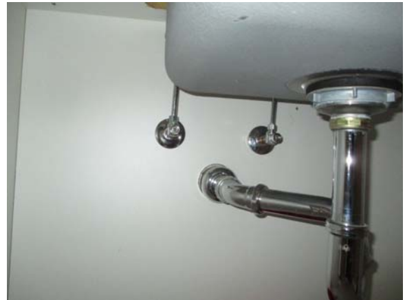
255029e 5/11/2021 Supply and drain piping Break room 2611C
