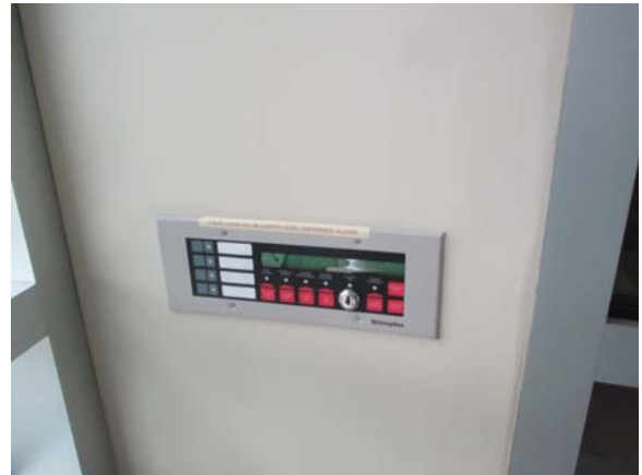
255041e 5/11/2021 Simplex remote annunciator for the FACP Southeast first floor entrance
