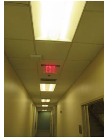
255025e 5/11/2021 2x4 lay-in fluorescent light fixtures Second floor corridor
