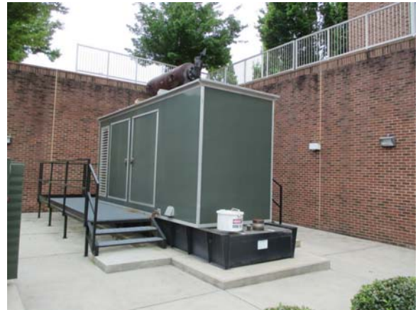
255065e 5/11/2021 250 kW diesel-fired generator sitting atop 750 gallon diesel tank North exterior
