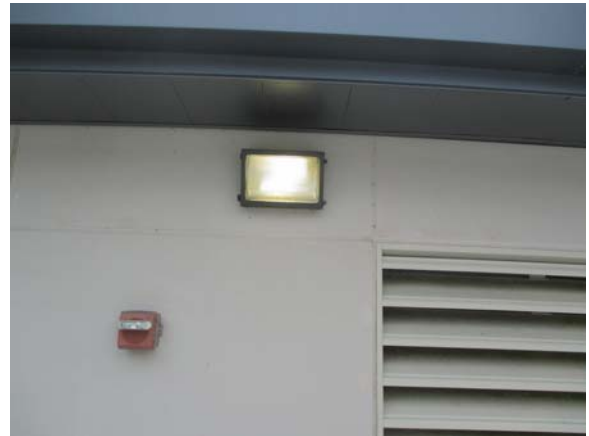
255005e 5/11/2021 Wall-mounted exterior light fixture and audible/visible fire device Center roof
