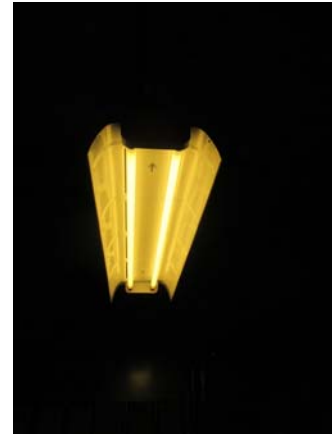
255010e 5/11/2021 Pendant fluorescent light fixture East penthouse
