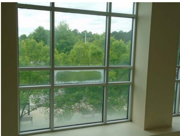
255048a 5/11/2021 Window condensation due to loss of seal Second floor
