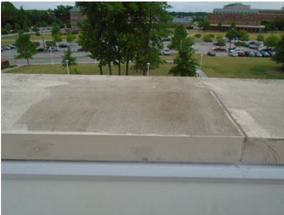
255020a 5/11/2021 Parapet cap is stained and damaged EIFS Roof
