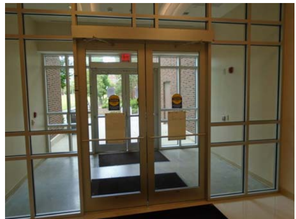
255099a 5/11/2021 Powered dual double doors with airlock First floor, north entrance
