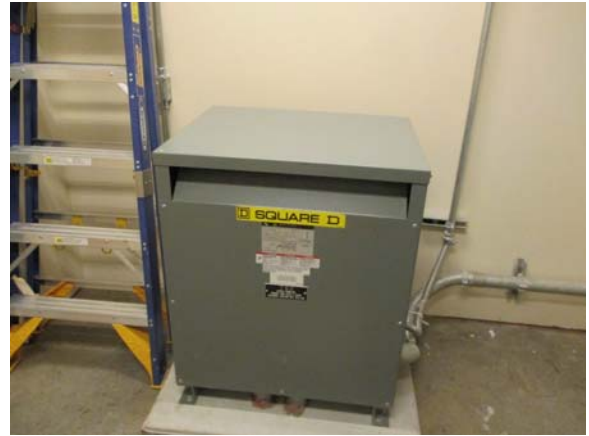
255022e 5/11/2021 112.5 kVA step-down Square D branch transformer Electrical room 2906A
