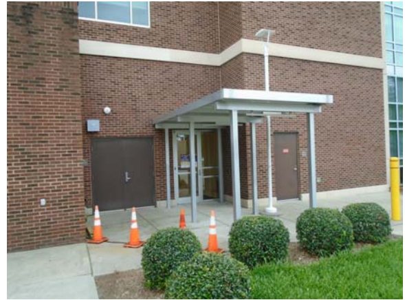
255119a 5/11/2021 Brick masonry, EIFS accents, and hollow metal service doors North exterior
