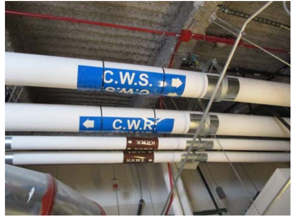
255007e 5/11/2021 Insulated piping with chilled water and heating hot water East penthouse
