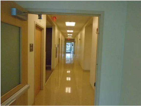
255070a 5/11/2021 Vinyl tile floor, painted walls, and suspended grid ceiling First floor corridor
