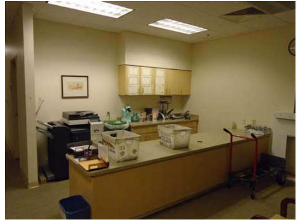
255107a 5/11/2021 Carpeting, painted walls and suspended grid ceiling Lower level office support area
