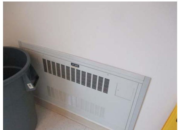
255042e 5/11/2021 Cabinet unit heater CUH-1922B First floor, north entrance
