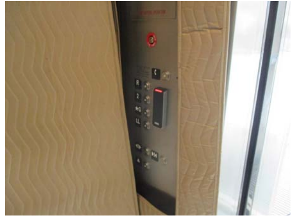
255001e 5/11/2021 Elevator control panel inside the service elevator Service elevator cab
