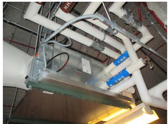
255012e 5/11/2021 Fan coil unit FCU-P-5 provides cooling and heating to the penthouse East penthouse
