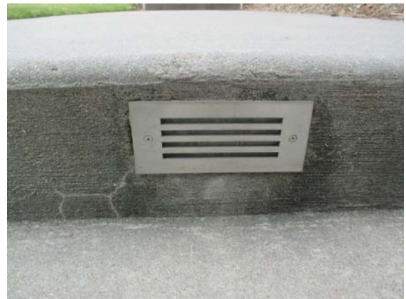
255075e 5/11/2021 Recessed step light North exterior
