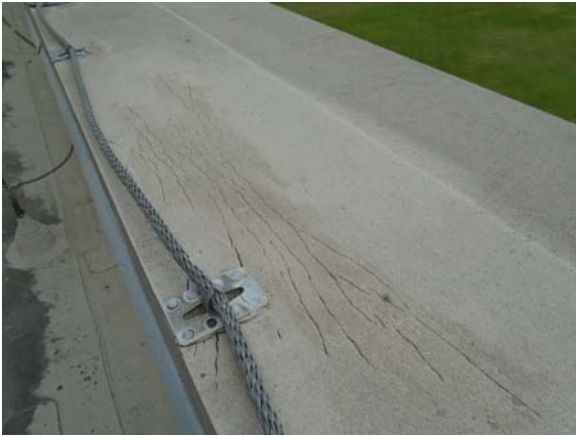
255022a 5/11/2021 Parapet cap is stained and damaged EIFS Roof
