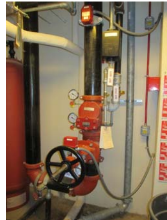
255050e 5/11/2021 Fire standpipe riser Room L914B
