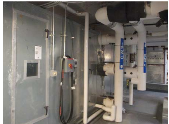
255015e 5/11/2021 Air handling unit AHU-5 with chilled water piping East penthouse
