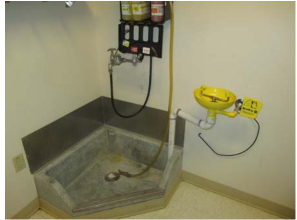
255037e 5/11/2021 Emergency eyewash station adjacent to service sink in custodial closet Room 2124B
