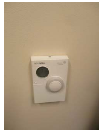
255024e 5/11/2021 Johnson Controls thermostat Electrical room 2906A
