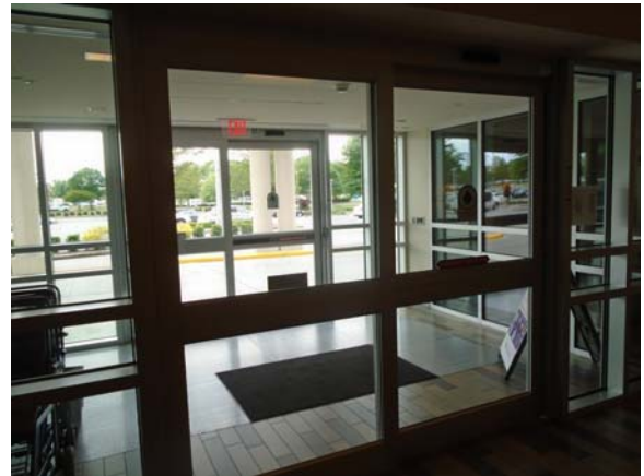
255085a 5/11/2021 Automatic double airlock glazed doorway system First floor lobby
