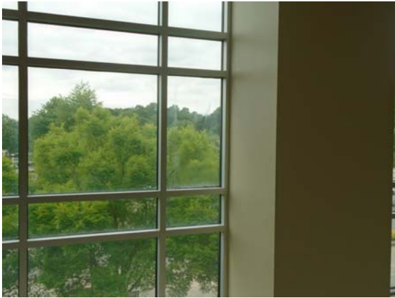
255049a 5/11/2021 Window condensation due to loss of seal Second floor
