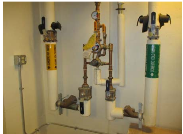
255051e 5/11/2021 Leonard mixing valve for domestic cold/hot water Room L914B
