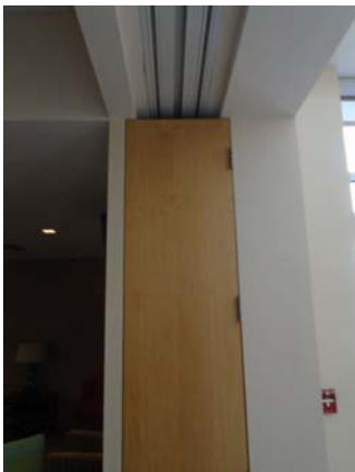
255086a 5/11/2021 Hidden fire door/curtain system around the atrium First floor lobby
