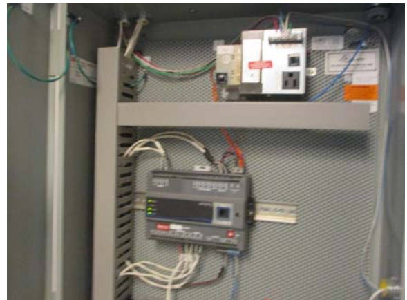
255018e 5/11/2021 Metasys controls for HVAC (FCU-3921) in the service elevator mechanical room Penthouse room 3921A
