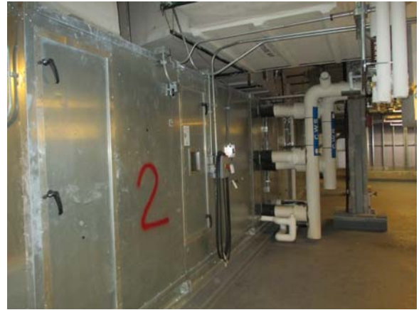
255019e 5/11/2021 Air handling unit AHU-2 with chilled water piping Southwest penthouse
