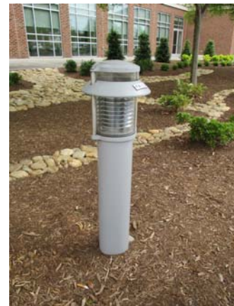
255072e 5/11/2021 Post-mounted LED light fixture South exterior
