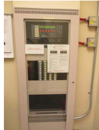
255064e 5/11/2021 Simplex fire alarm control panel Lower level service entry
