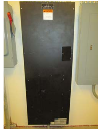
255023e 5/11/2021 Lutron lighting control panel Electrical room 2906A
