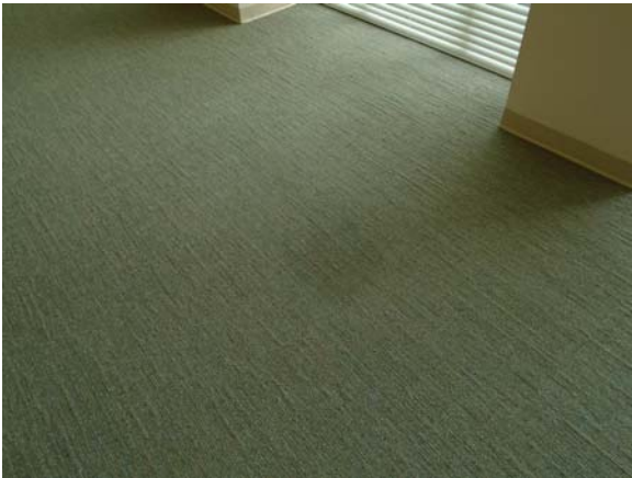
255032a 5/11/2021 Stained carpet Second floor student lounge
