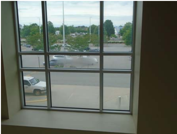
255047a 5/11/2021 Window condensation due to loss of seal Second floor
