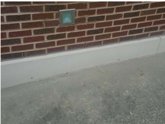
255128a 5/11/2021 Screws visible in EIFS panels West exterior
