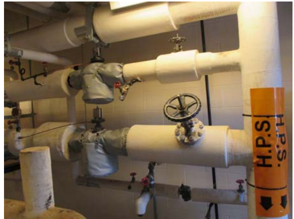
255056e 5/11/2021 Spirax Sarco steam pressure reducing valves Room L914B
