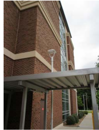
255068e 5/11/2021 15 foot stanchion LED light fixture North exterior
