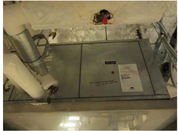
255061e 5/11/2021 Fan coil unit FCU-L-914B that cools and heats basement mechanical room Room L914B
