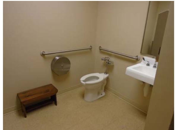
255103a 5/11/2021 Accessible fixtures and vinyl floor tile Lower level single-user restroom
