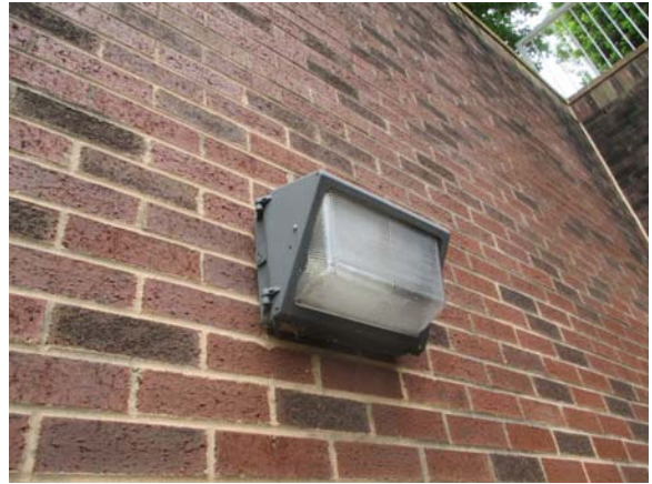
255067e 5/11/2021 Wall-mounted CFL exterior light fixture North exterior
