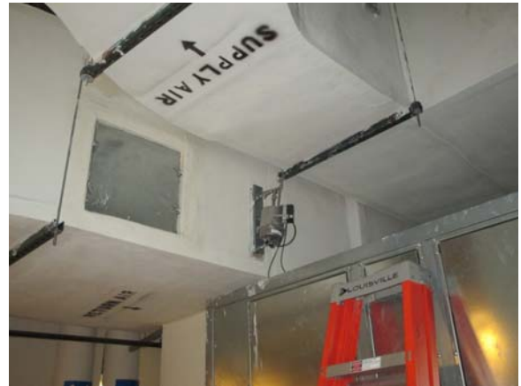
255014e 5/11/2021 Pneumatic actuator on the return air ductwork for AHU-5 East penthouse
