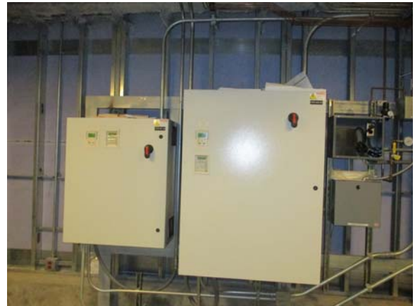
255011e 5/11/2021 Two variable frequency drives for AHU-3 supply and return fans East penthouse
