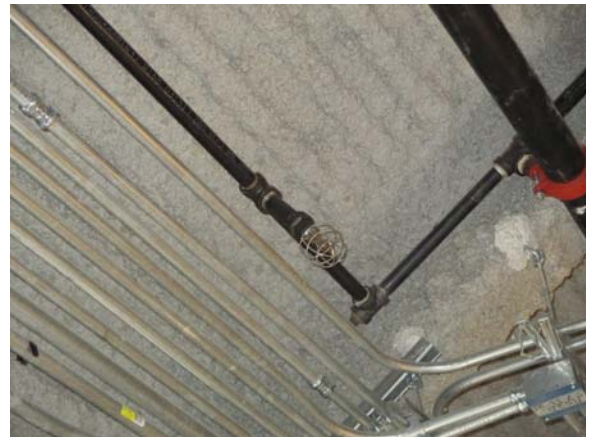
255006e 5/11/2021 Sprinkler head East penthouse
