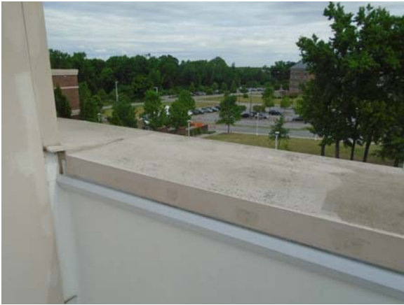
255019a 5/11/2021 Parapet cap is stained EIFS Roof
