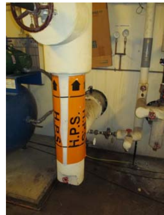
255054e 5/11/2021 Insulated high pressure steam piping entering the building Room L914B
