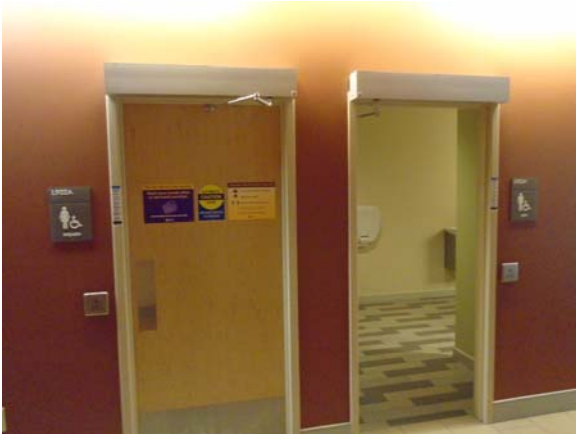
255108a 5/11/2021 Power door operators on restrooms Lower level
