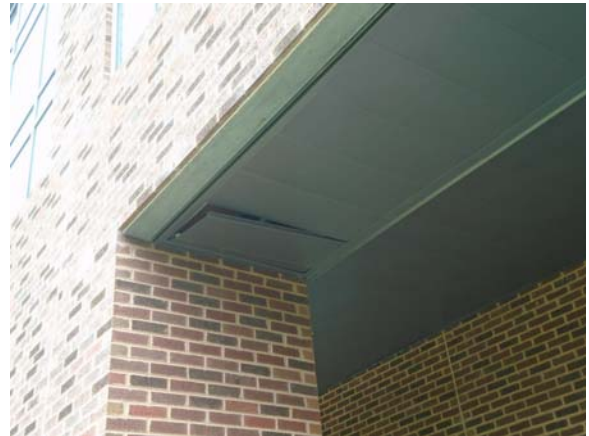
255127a 5/11/2021 Metal fascia needing repair West exterior
