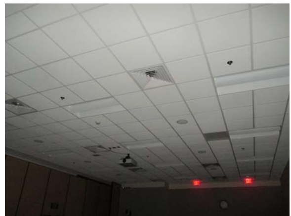
255030e 5/11/2021 Lighting Large meeting room 2610C
