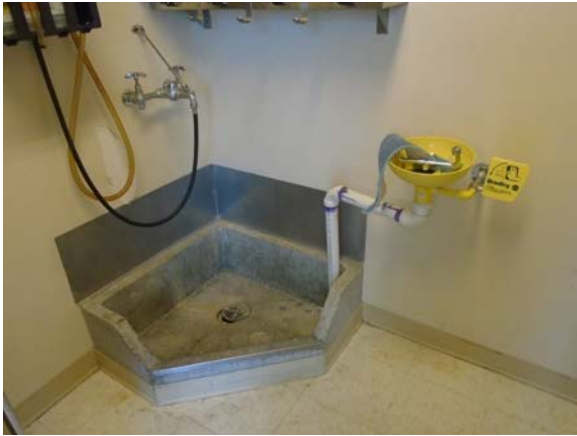
255094a 5/11/2021 Utility floor sink with emergency eyewash First floor janitorial closet
