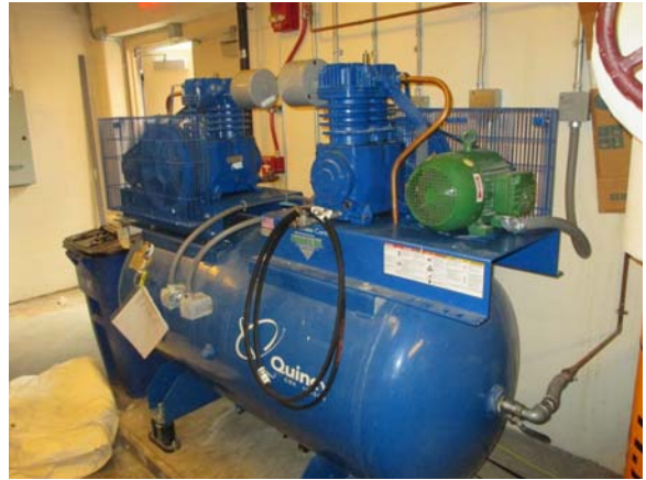
255055e 5/11/2021 Quincy air compressor for HVAC pneumatic controls Room L914B
