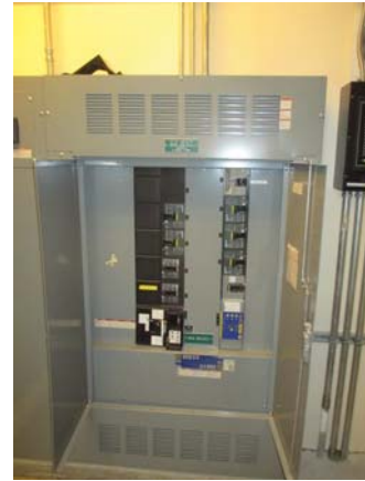
255049e 5/11/2021 Square D 400 amp generator switchboard G2-MDP Room L907B
