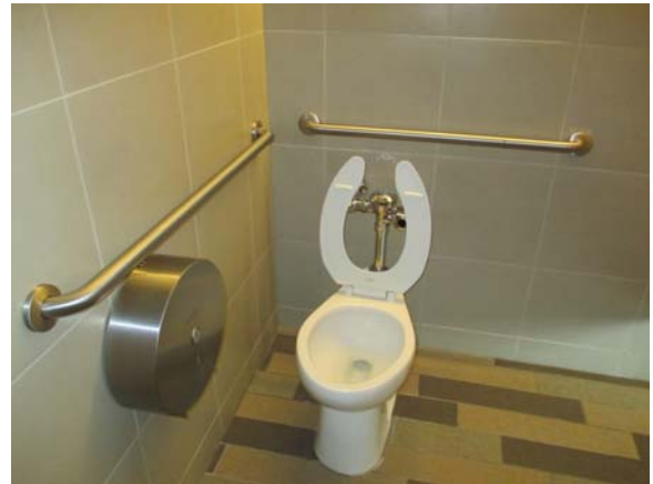
255035e 5/11/2021 Hands-free water closet Men's restroom 2903A
