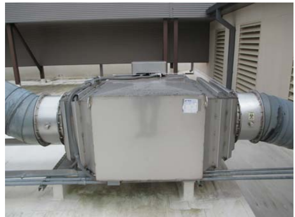
255003e 5/11/2021 HEPA filter connected to EF-1A and EF-1B ductwork Center roof
