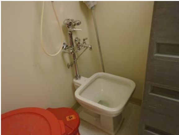
255096a 5/11/2021 Ceramic pedestal floor basin First floor biohazard room
