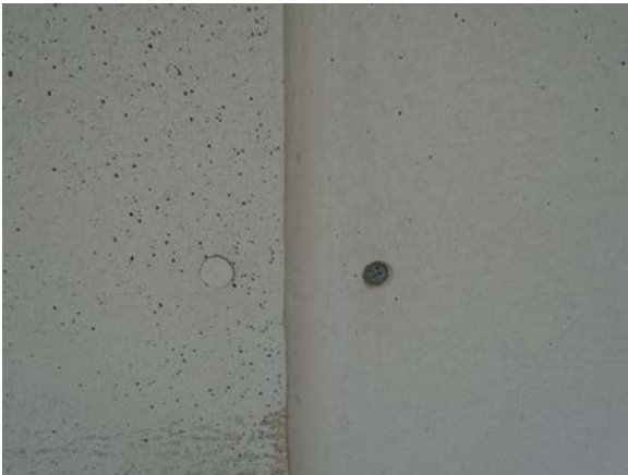
255014a 5/11/2021 Screws visible in panels Mechanical penthouse
