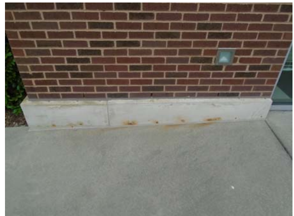
255141a 5/11/2021 Screws rusting in EIFS accents Northeast exterior
