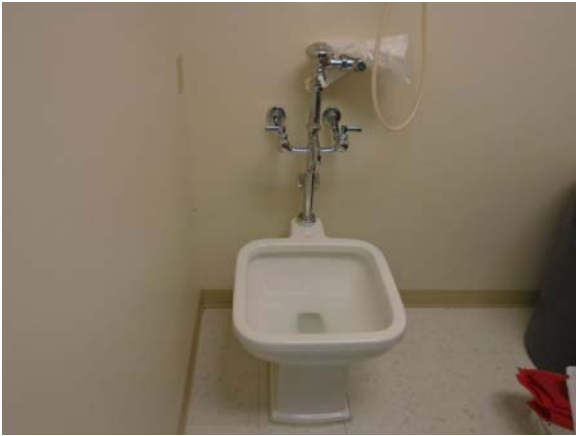
255073a 5/11/2021 Ceramic pedestal floor basin Biohazard room 1803C
