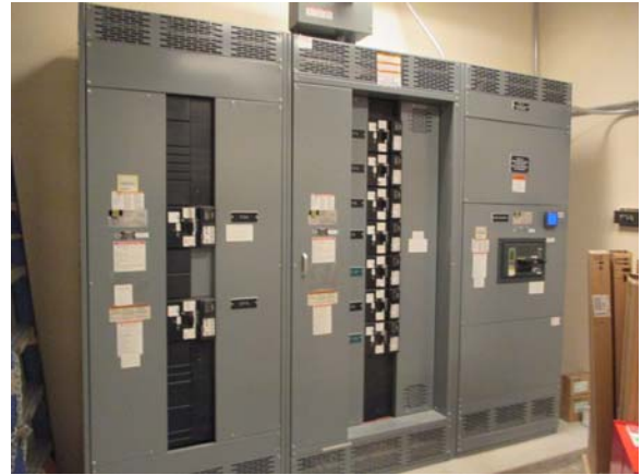
255046e 5/11/2021 Square D 2,000 amp main distribution panel Room L906B
