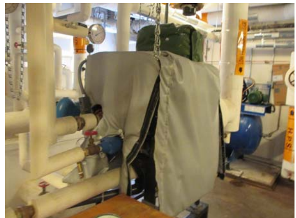
255063e 5/11/2021 Domestic hot water is produced by heat exchanger under the insulating jacket Room L914B
