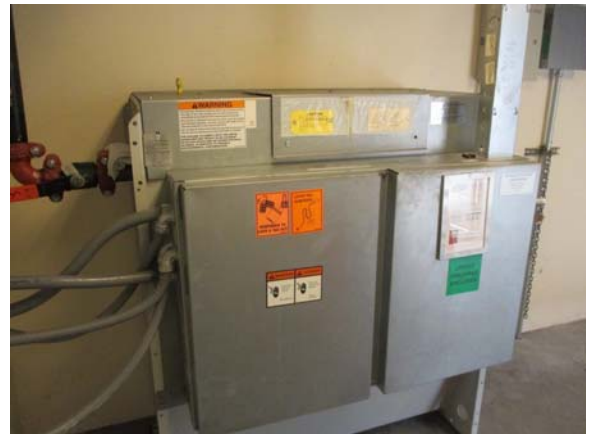
255017e 5/11/2021 Hydraulic pump and controls for the Schindler service elevator Penthouse room 3921A
