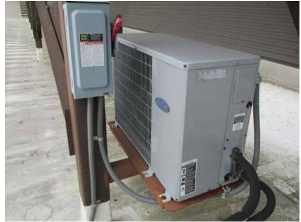
255004e 5/11/2021 1.5 ton Carrier condensing unit Center roof
