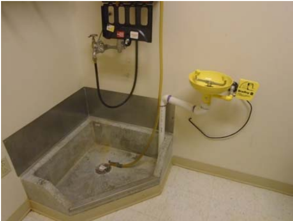
255064a 5/11/2021 Utility floor sink with emergency eyewash Janitorial closet 2124B
