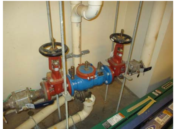
255053e 5/11/2021 One of three 2 inch backflow preventers Room L914B
