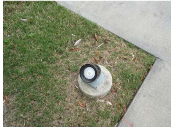
255073e 5/11/2021 Ground-mounted LED light fixture South exterior
