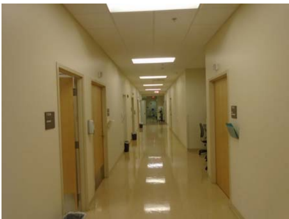
255080a 5/11/2021 Vinyl tile floor, painted walls, and suspended grid ceiling First floor corridor
