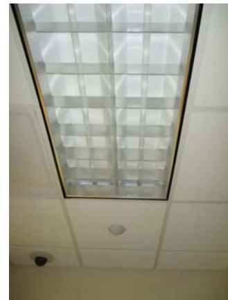
255033e 5/11/2021 2x4 lay-in fluorescent light fixtures Counseling room 2302A
