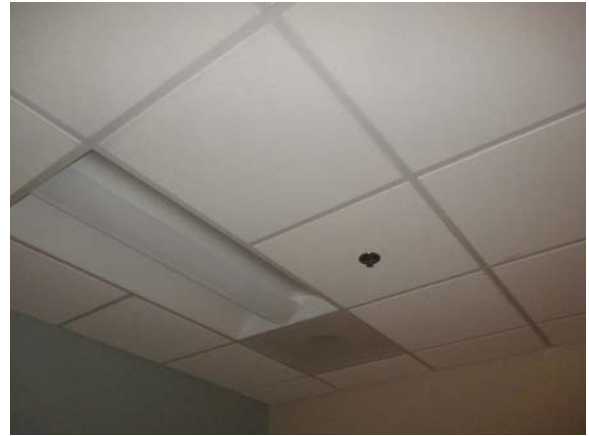
255040e 5/11/2021 2x4 fluorescent light fixture in typical exam room Room 1412C
