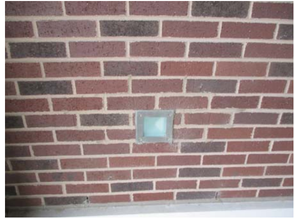
255070e 5/11/2021 Square recessed LED light fixture West exterior
