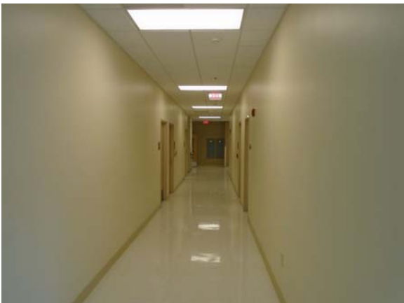
255072a 5/11/2021 Vinyl tile floor, painted walls, and suspended grid ceiling First floor corridor
