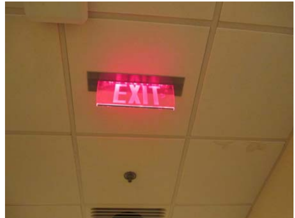
255026e 5/11/2021 Edge-lit LED exit sign Second floor corridor
