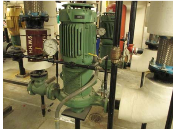
255058e 5/11/2021 15 hp HWP-1 heating hot water pump Room L914B
