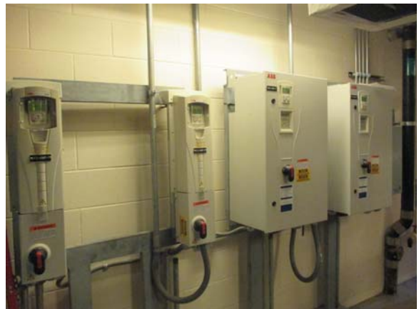
255057e 5/11/2021 Four variable frequency drives controlling hot water and chilled water pumps Room L914B
