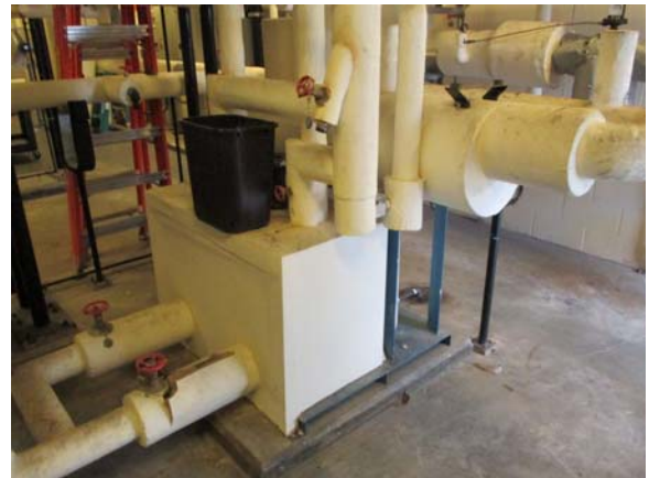
255062e 5/11/2021 Pneumatic condensate receiver Room L914B
