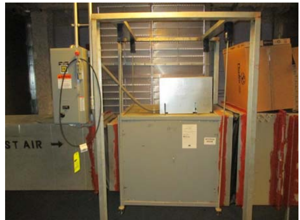
255021e 5/11/2021 5 hp exhaust fan EF-2 Southwest penthouse
