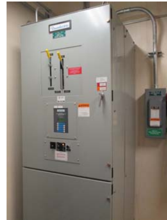
255047e 5/11/2021 Russelectric 600 amp automatic transfer switch ATS-G1 Room L907B
