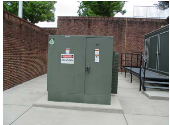
255066e 5/11/2021 1,000 amp oil-filled primary transformer North exterior
