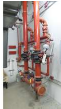
AHSB035e 4/20/2016 Wet-pipe fire system risers #1 and #2 Room 1510B
