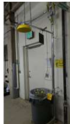
AHSB036e 4/20/2016 Combination emergency shower and eyewash station Room 1510B
