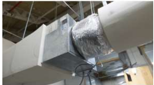
AHSB051e 4/20/2016 Variable air volume terminal Penthouse D
