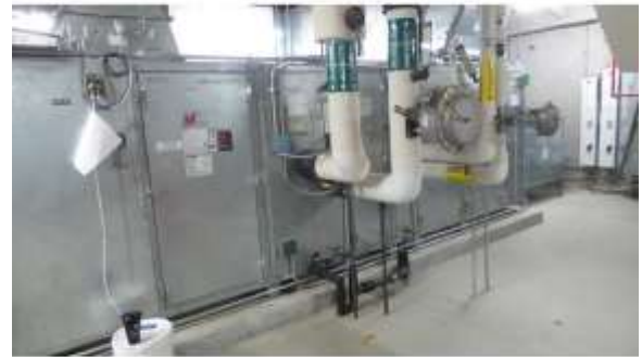
AHSB008e 4/20/2016 Air handler AHU-3E East penthouse
