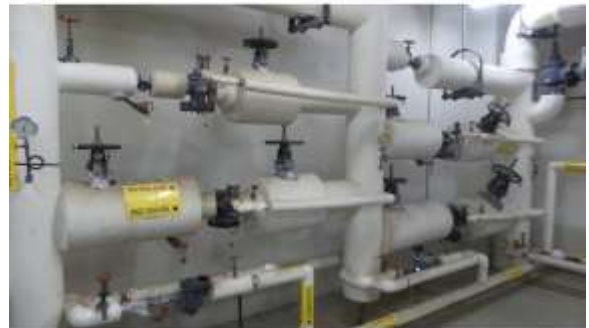
AHSB023e 4/20/2016 Pressure reducing valve systems Room 1510B
