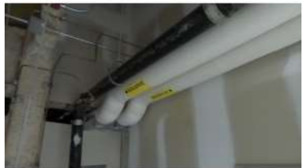
AHSB012e 4/20/2016 Heating water supply and return and waste water piping East penthouse
