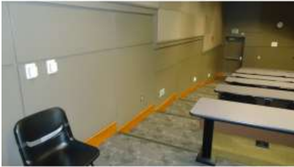
AHSB040a 4/20/2016 Terraced classroom without handrails along the outer wall First floor, north
