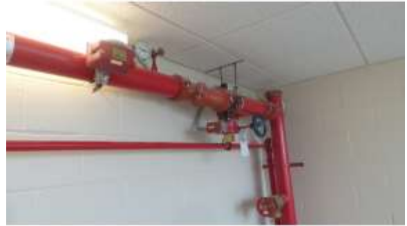
AHSB016e 4/20/2016 Fire riser with tamper switch and control valves Fifth floor, stairwell 6
