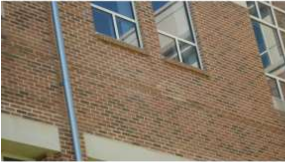
AHSB052a 4/20/2016 Deficient exterior brick masonry and a previous repair Exterior envelope
