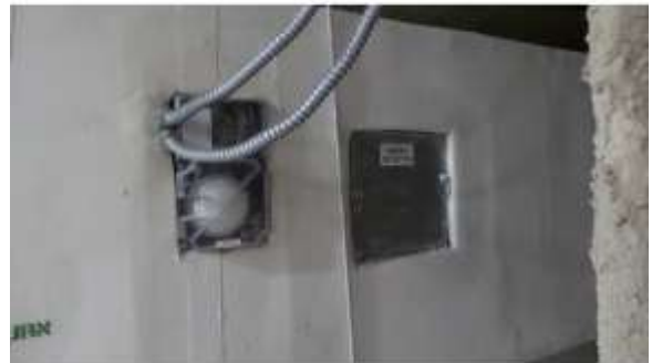
AHSB003e 4/20/2016 Duct-mounted smoke detector East penthouse
