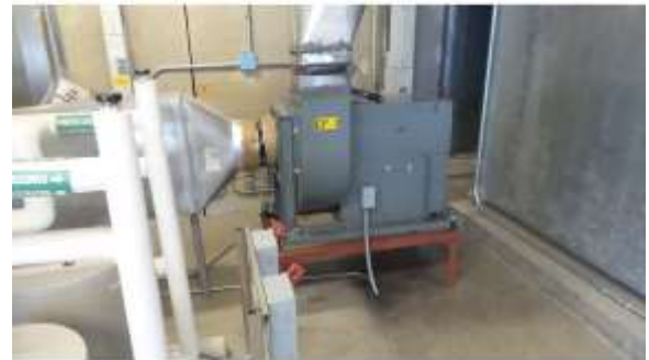
AHSB048e 4/20/2016 Utility set exhaust fan EF-1 Penthouse B
