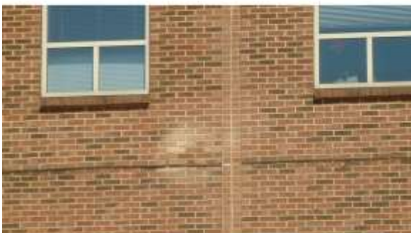
AHSB075a 4/20/2016 Deficient exterior brick masonry and a previous repair Exterior envelope
