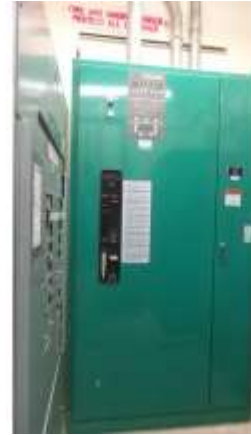
AHSB044e 4/20/2016 Automatic transfer switch ATS EQ Room 1514
