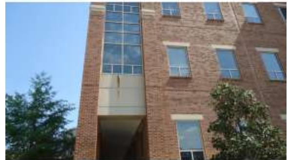
AHSB080a 4/20/2016 Corrosion stain on exterior concrete veneer Exterior envelope
