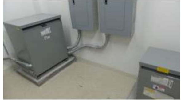
AHSB022e 4/20/2016 Secondary electric system transformers and panelboards Room 4520
