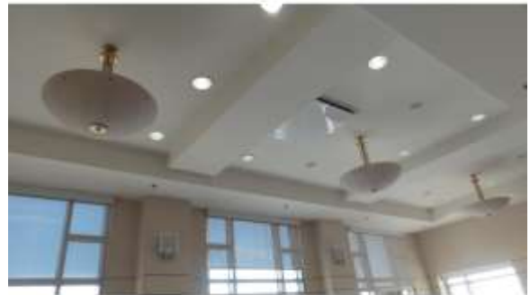
AHSB018e 4/20/2016 Various elegant, sconce, and recessed lighting Fourth floor, common space near terrace
