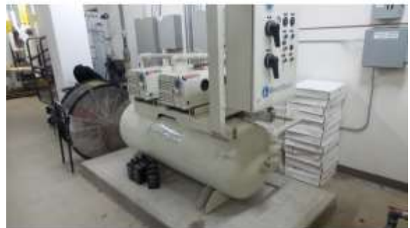
AHSB039e 4/20/2016 Laboratory duplex vacuum pump system Room 1510B
