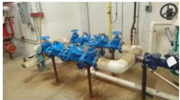
AHSB033e 4/20/2016 Two double-check, domestic water backflow preventers Room 1510B
