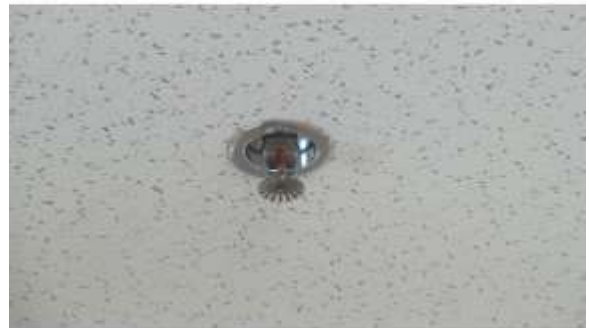
AHSB021e 4/20/2016 Typical glass bulb fire system sprinkler head Room 4508
