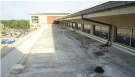
AHSB003a 4/20/2016 Single-ply TPO, flat roof and pitched standing seam metal roof Upper level roof
