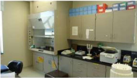
AHSB032a 4/20/2016 Vinyl tiled floors, suspended grid ceilings, and lab cabinetry Fourth floor, northern lab
