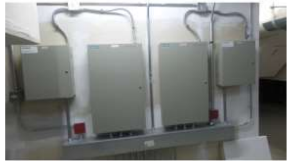
AHSB014e 4/20/2016 Various direct digital and pneumatic control panels East penthouse
