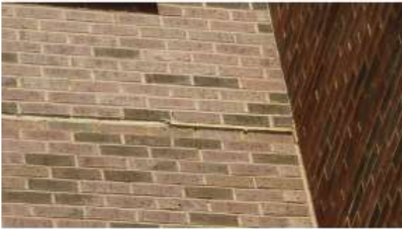
AHSB056a 4/20/2016 Deficient exterior brick masonry and a previous repair Exterior envelope
