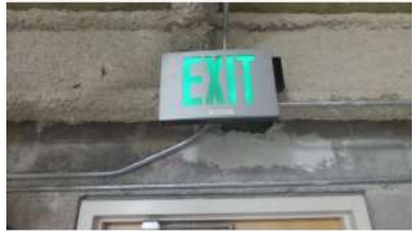
AHSB002e 4/20/2016 Typical exit signage East penthouse
