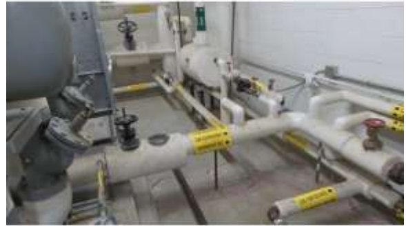
AHSB031e 4/20/2016 Various condensate return piping systems Room 1510B
