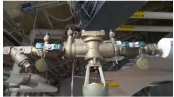
AHSB010e 4/20/2016 One-inch backflow preventer East penthouse
