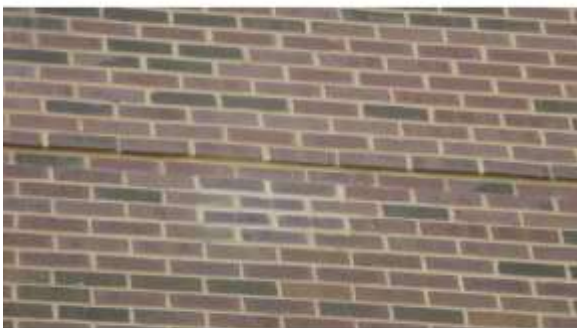
AHSB063a 4/20/2016 Deficient exterior brick masonry and a previous repair Exterior envelope
