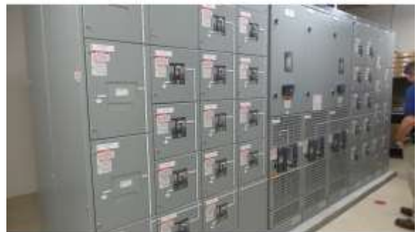
AHSB042e 4/20/2016 3,200 amp low-voltage circuit breaker switchgear Room 1514
