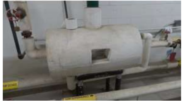
AHSB025e 4/20/2016 Flash tank #1 Room 1510B
