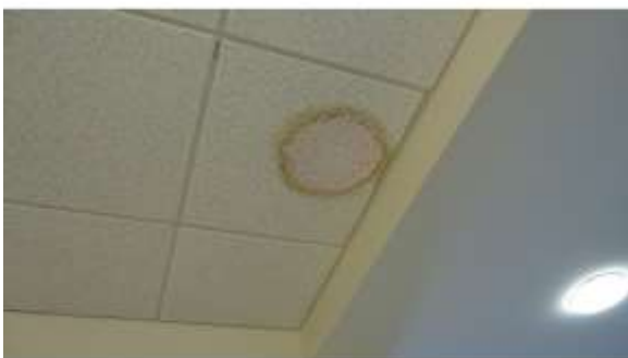
AHSB036a 4/20/2016 Ceiling tile water stained from fire suppression system Second floor
