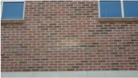
AHSB071a 4/20/2016 Deficient exterior brick masonry and a previous repair Exterior envelope
