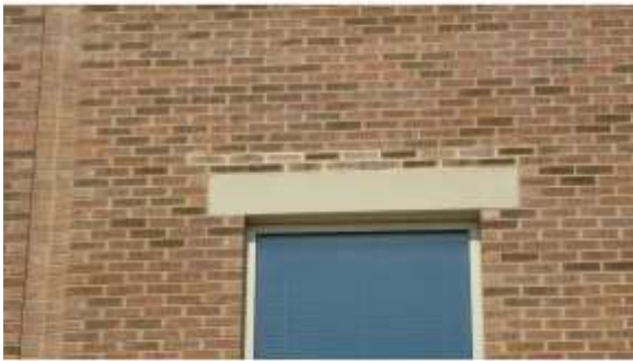
AHSB085a 4/20/2016 Deficient exterior brick masonry and a previous repair Exterior envelope
