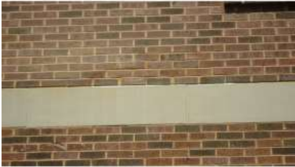
AHSB059a 4/20/2016 Deficient exterior brick masonry and a previous repair Exterior envelope
