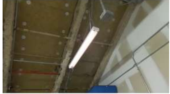
AHSB001e 4/20/2016 Interior light fixture East penthouse
