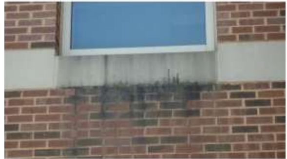
AHSB070a 4/20/2016 Stained and deficient exterior brick masonry Exterior envelope
