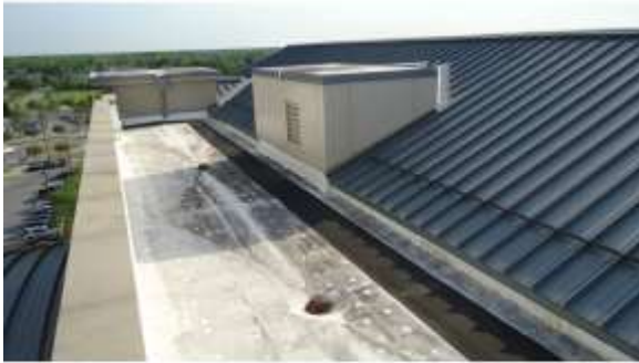
AHSB004a 4/20/2016 Single-ply TPO, flat roof and pitched standing seam metal roof Upper level roof
