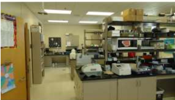
AHSB033a 4/20/2016 Vinyl tiled floors, suspended grid ceilings, and metal lab cabinetry Fourth floor, northern lab
