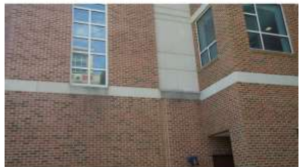
AHSB064a 4/20/2016 Stained and deficient exterior brick masonry Exterior envelope
