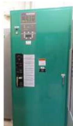
AHSB045e 4/20/2016 Automatic transfer switch ATS LS Room 1514
