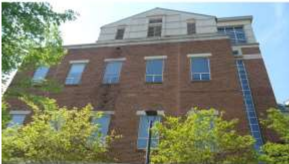
AHSB045a 4/20/2016 Stained exterior brick masonry Exterior envelope
