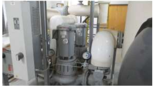
AHSB029e 4/20/2016 Heating water pumps HWP-1 and HWP-2 Room 1510B
