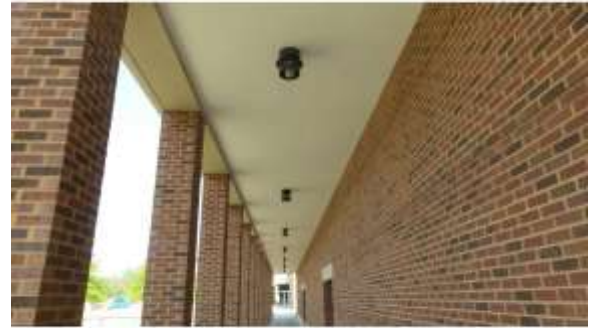
AHSB055e 4/20/2016 Surface-mounted exterior light fixtures Exterior
