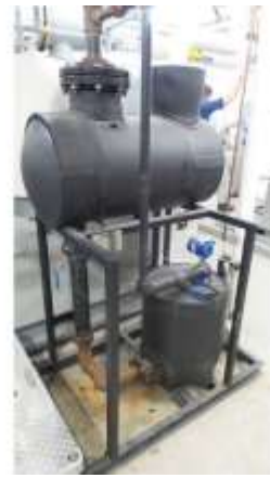
AHSB028e 4/20/2016 Vacuum condensate return skid Room 1510B
