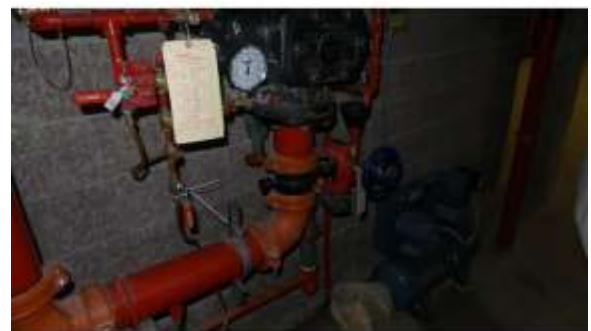
AHSB015e 4/20/2016 Preaction fire system air compressor East penthouse
