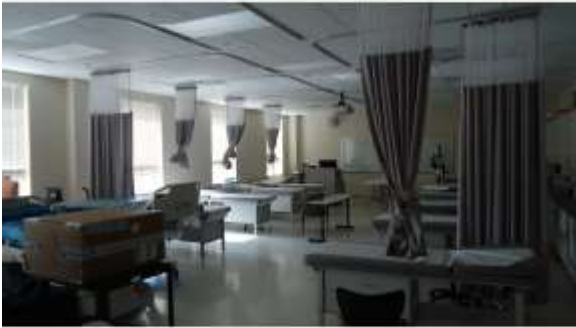
AHSB031a 4/20/2016 Vinyl tiled floors and suspended grid ceilings Fourth floor, teaching lab
