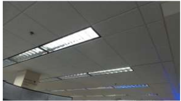
AHSB017e 4/20/2016 Recessed, 1x4 fluorescent lighting with T8 lamps Fourth floor, common space near 4508
