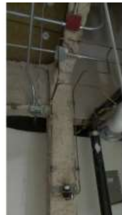
AHSB013e 4/20/2016 Pneumatic control system piping East penthouse
