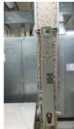
AHSB006e 4/20/2016 Variable frequency drive AHU-3E East penthouse
