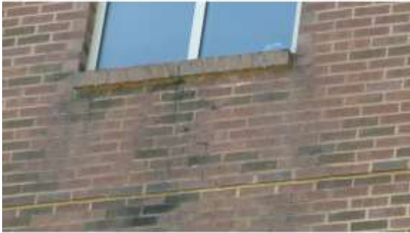
AHSB046a 4/20/2016 Stained and deficient exterior brick masonry Exterior envelope
