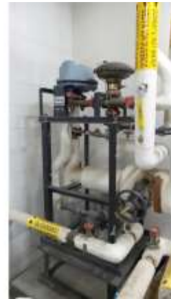
AHSB026e 4/20/2016 Unfired domestic water heating skid DWH-1 Room 1510B
