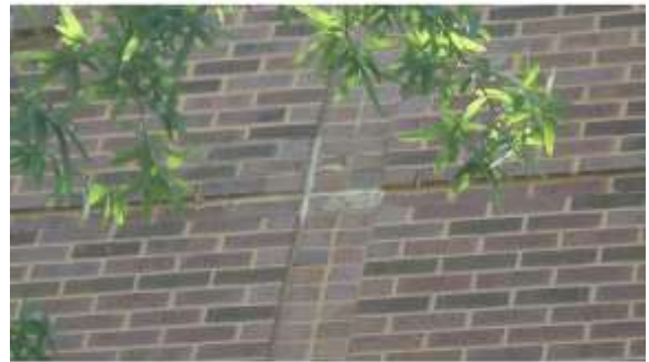
AHSB062a 4/20/2016 Deficient exterior brick masonry and a previous repair Exterior envelope
