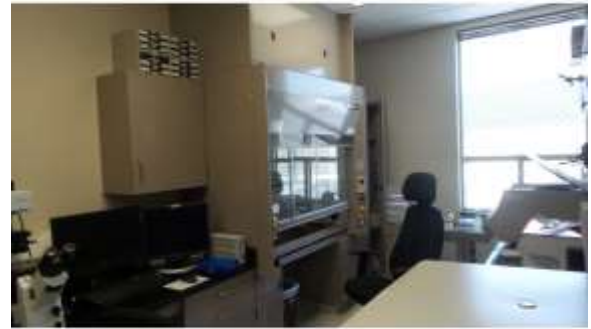
AHSB047e 4/20/2016 Fume hood FH-4165-1 Room 4165B
