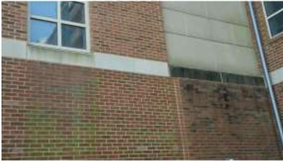
AHSB049a 4/20/2016 Stained and deficient exterior brick masonry Exterior envelope
