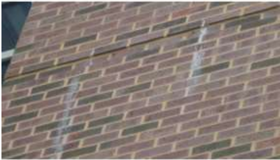
AHSB047a 4/20/2016 Stained and deficient exterior brick masonry Exterior envelope
