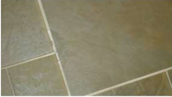
AHSB043a 4/20/2016 Chipped slate floor tile First floor, north
