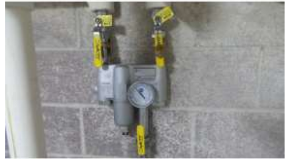
AHSB053e 4/20/2016 Dedicated mixing valve for emergency plumbing fixture Penthouse D
