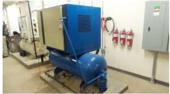
AHSB040e 4/20/2016 Control systems air compressor Room 1510B
