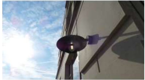
AHSB019e 4/20/2016 Exterior sconce fixture with CFL lamp Fourth floor, terrace
