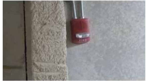
AHSB007e 4/20/2016 Fire alarm system device with visual and audible annunciation East penthouse
