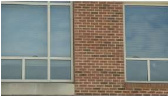
AHSB073a 4/20/2016 Rubber gasket seal coming out in interior West elevation, A wing
