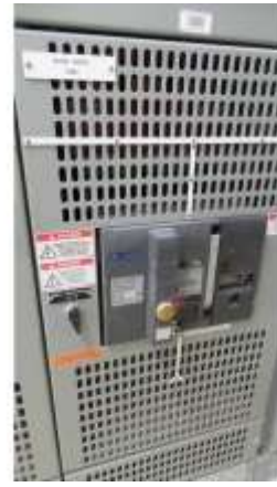
AHSB043e 4/20/2016 Power circuit breaker main MSB1 Room 1514
