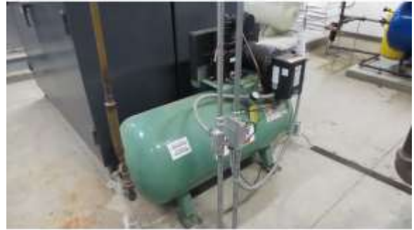
AHSB037e 4/20/2016 Pumped condensate air compressor Room 1510B
