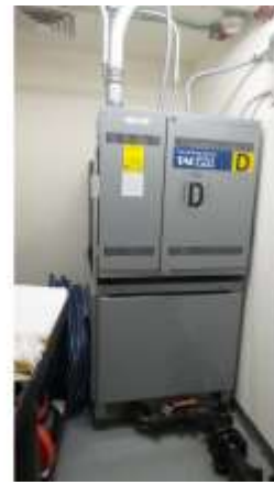
AHSB046e 4/20/2016 Hydraulic elevator machine D Room 1427
