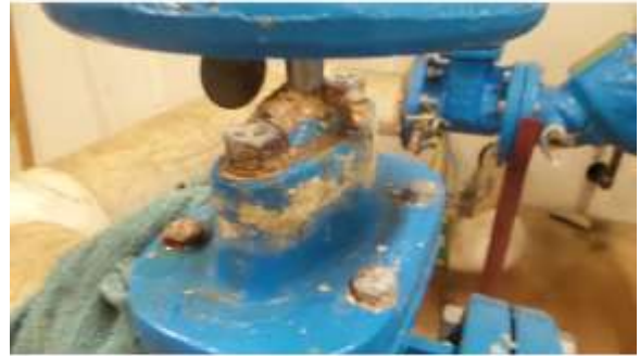
AHSB034e 4/20/2016 Minor calcification of the DW BFP valve stem Room 1510B
