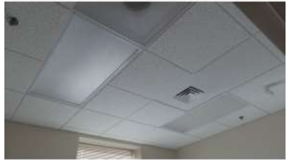
AHSB020e 4/20/2016 Recessed, 2x4 foot fluorescent lighting with T8 lamps Room 4508
