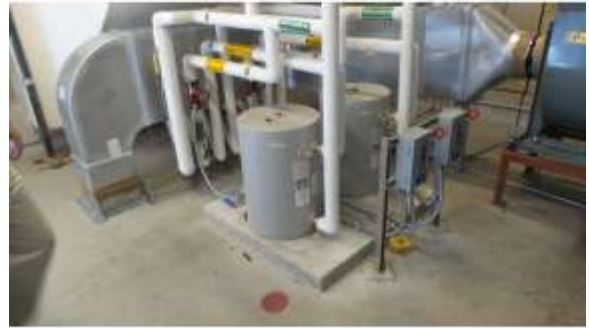
AHSB049e 4/20/2016 Two electric water heaters Penthouse B
