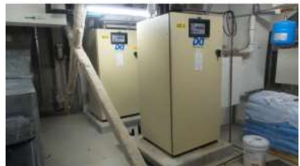
AHSB009e 4/20/2016 18 ton computer room air conditioner East penthouse
