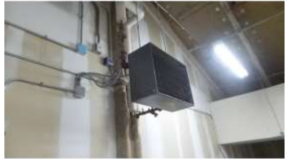
AHSB004e 4/20/2016 Hydronic unit heater East penthouse
