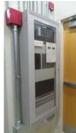
AHSB041e 4/20/2016 Point addressable fire alarm control panel Room 1514
