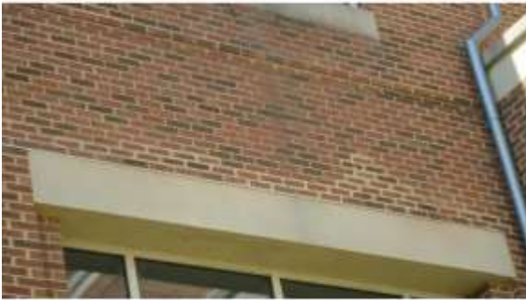
AHSB053a 4/20/2016 Deficient exterior brick masonry and a previous repair Exterior envelope
