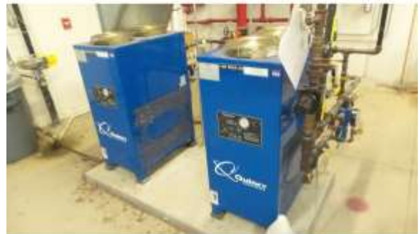
AHSB038e 4/20/2016 Air dryers #1 and #2 Room 1510B
