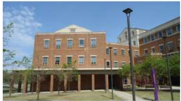
AHSB074a 4/20/2016 Brick masonry, dual-pane or tempered glazing, and standing seam metal roof East elevation, A wing
