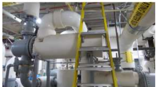
AHSB030e 4/20/2016 Shell-and-tube heat exchanger PHE-1 Room 1510B
