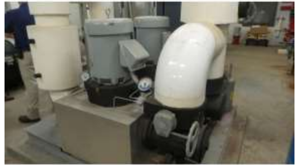
AHSB032e 4/20/2016 Chilled water pumps CHWP-1 and CHWP-2 Room 1510B
