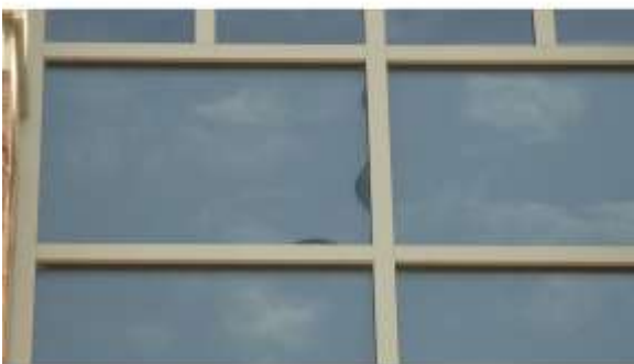
AHSB081a 4/20/2016 Rubber gasket seal coming out in interior South elevation, E wing
