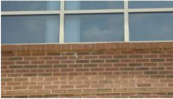
AHSB083a 4/20/2016 Deficient exterior brick masonry and a previous weep repair Exterior envelope
