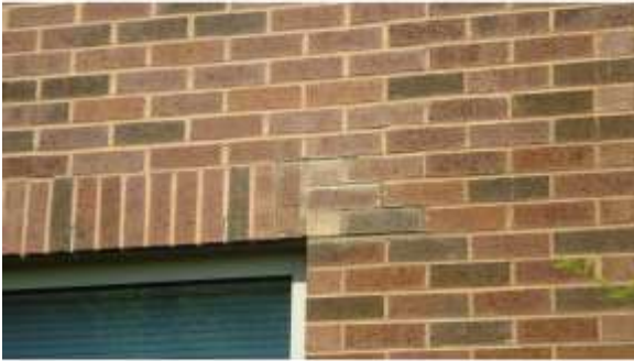
AHSB055a 4/20/2016 Deficient exterior brick masonry and a previous repair Exterior envelope
