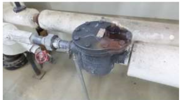
AHSB024e 4/20/2016 Steam trap Room 1510B
