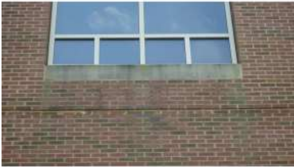
AHSB050a 4/20/2016 Stained and deficient exterior brick masonry Exterior envelope
