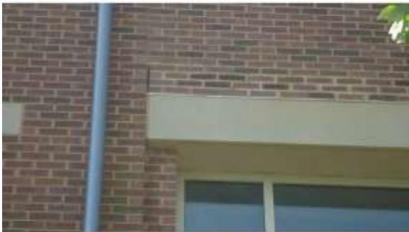
AHSB051a 4/20/2016 Previous masonry repair Exterior envelope
