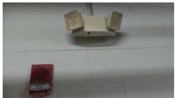
AHSB027e 4/20/2016 Twin, sealed emergency light fixture Room 1510B
