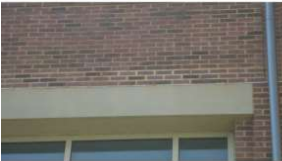
AHSB054a 4/20/2016 Deficient exterior brick masonry and a previous repair Exterior envelope
