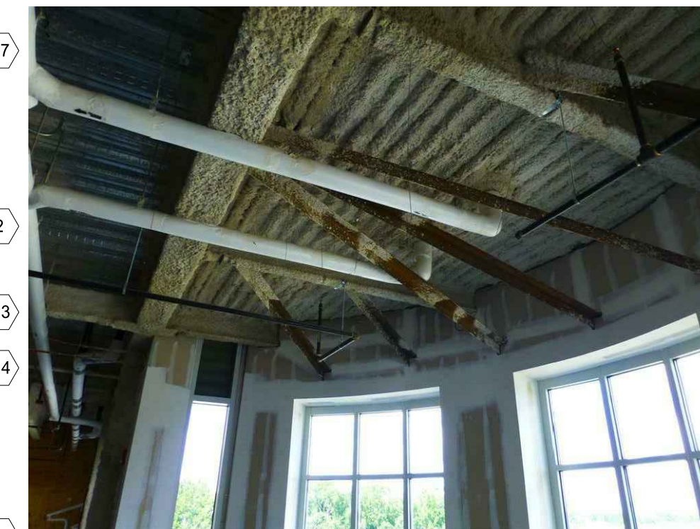
IMAGE B: EXISTING CEILING AND EXTERIOR WALL CONDITION IN CONFERENCE ROOM 4130.
