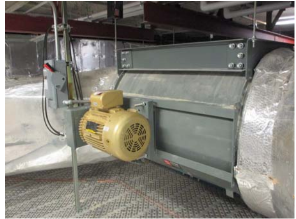
256037e 5/11/2021 25 hp return fan for the B side of AHU-CL-2 Penthouse
