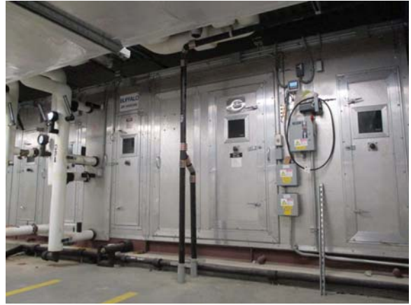
256129e 5/11/2021 Buffalo air handling unit (AHU-A-1) serving the lecture halls Room 3300
