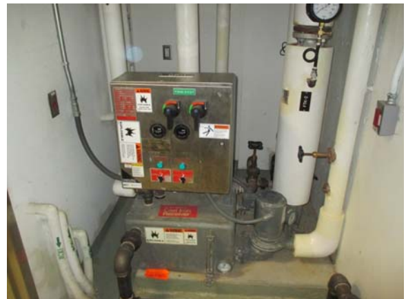
256105e 5/11/2021 Steam condensate receiver for sterilizers Room 1258
