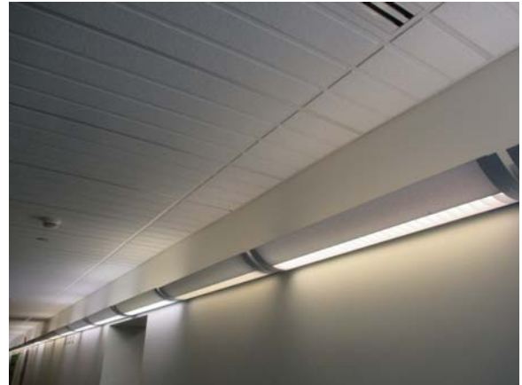
256079e 5/11/2021 Wall-mounted fluorescent light fixtures Third floor corridor
