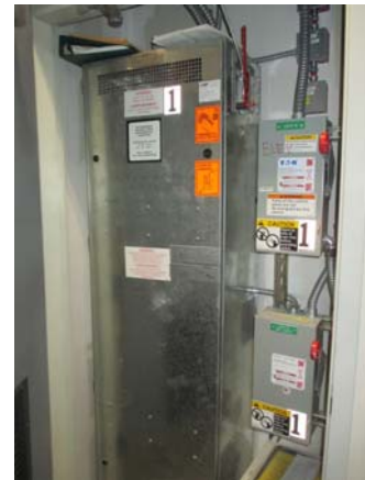
256027e 5/11/2021 Controls for the freight (traction) elevator Room 5104
