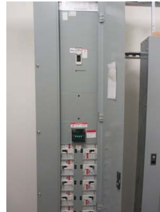
256014e 5/11/2021 480/277 volt Eaton secondary electrical panel Room 5103
