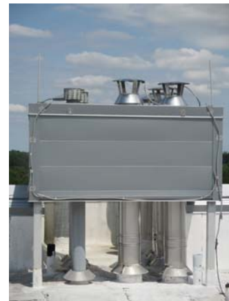
256012e 5/11/2021 Multiple exhaust stacks coming through the roof East end of roof
