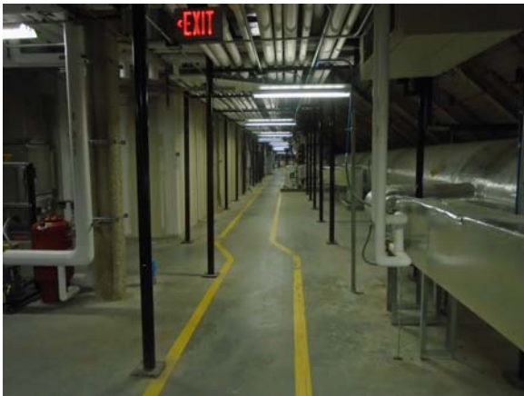
256041a 5/12/2021 Painted safety striping and adequate emergency exit signage Fifth floor mechanical attic
