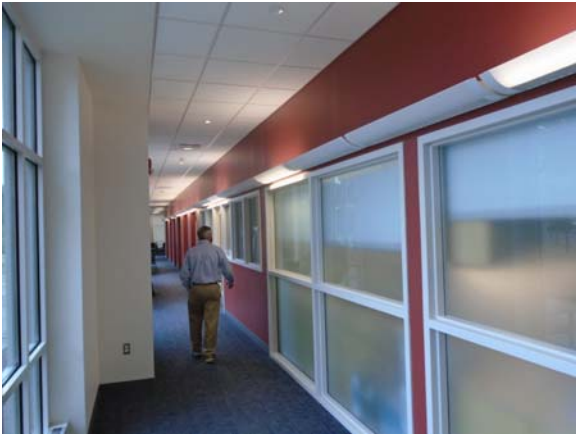
256092a 5/12/2021 Carpeting, painted walls, and suspended grid ceiling Second floor outer corridor
