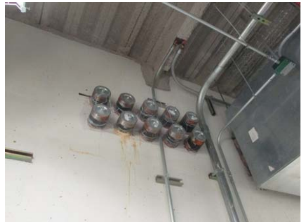
256101e 5/11/2021 Conduit has already been placed for the second 2,000 kVA oil-filled transformer Room E1182
