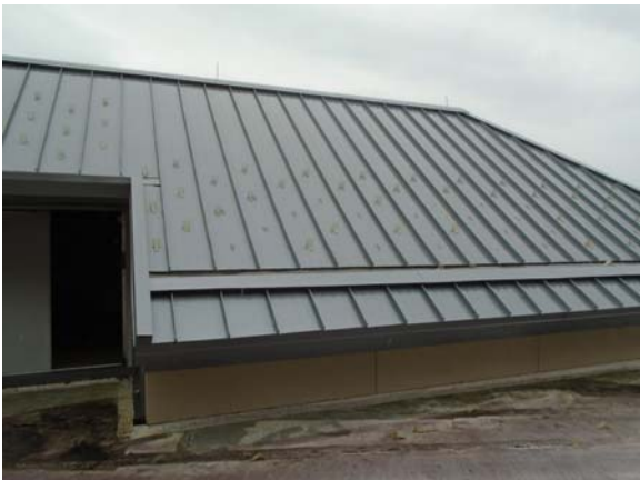
256126a 5/12/2021 Broken plastic "ice cleats" attached to metal roofing Pitched standing seam metal roof
