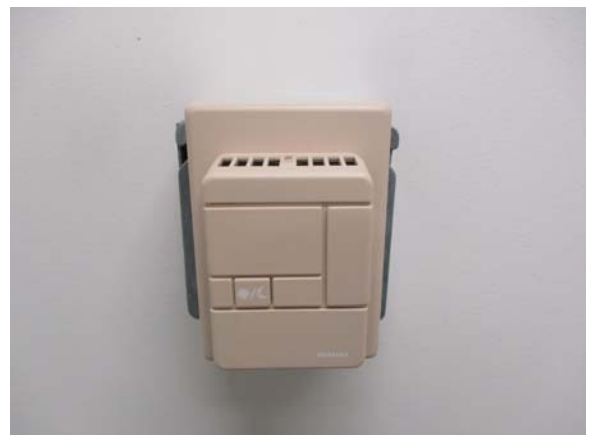
256015e 5/11/2021 Siemens thermostat for HVAC control Room 5103
