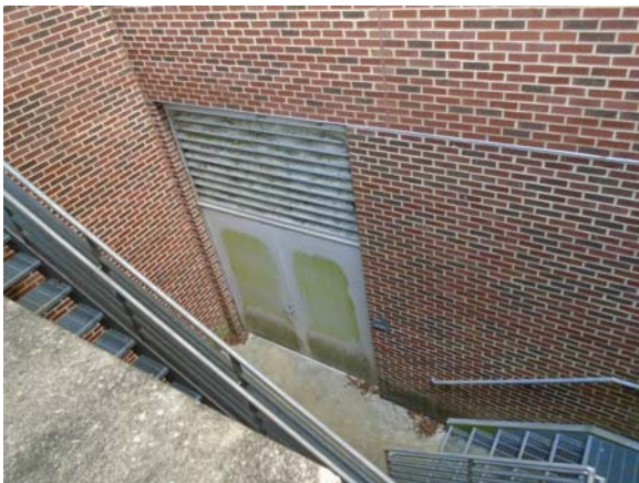
256012a 5/12/2021 Hollow metal service doors and vents with staining North exterior
