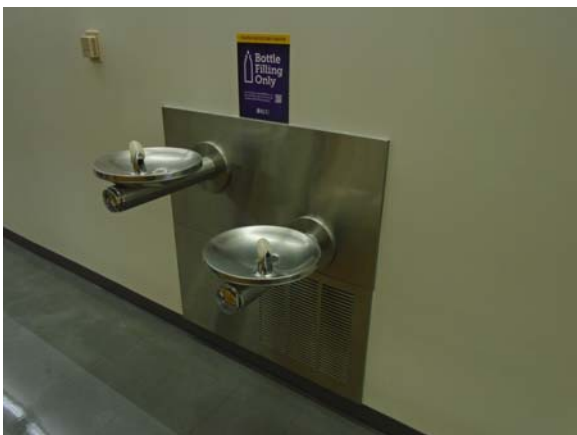
256099a 5/12/2021 Dual-level water fountain Second floor
