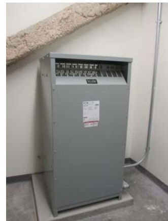
256072e 5/11/2021 Eaton dry-type step-down transformer Room 4101A
