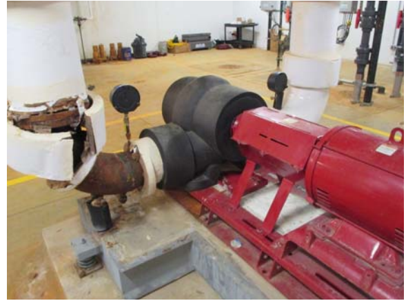
256122e 5/11/2021 40 hp CHP-1 chilled water pump Room B0100
