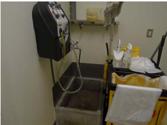
256072a 5/12/2021 Concrete molded floor sink Janitorial closet 4060
