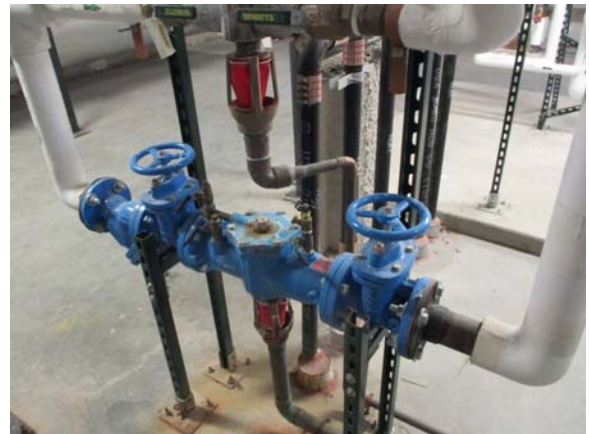
256047e 5/11/2021 3 inch backflow preventer on domestic water East end of penthouse
