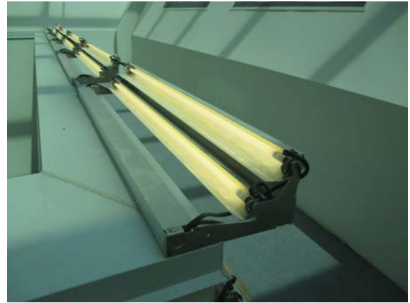
256016e 5/11/2021 T5 fluorescent light fixtures illuminating the top of the atrium Top of atrium
