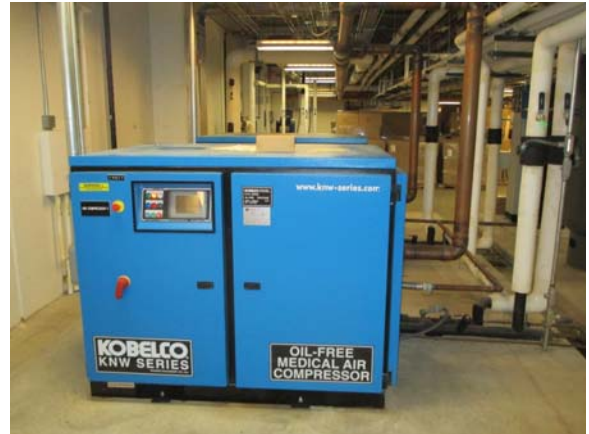
256124e 5/11/2021 One of two 75 hp Kobelco air compressor systems for dental and lab areas Room B0100
