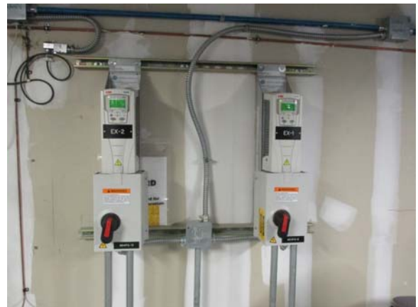
256024e 5/11/2021 Variable frequency drives (VFD) for EX-2 and EX-1 Northwest corner of penthouse
