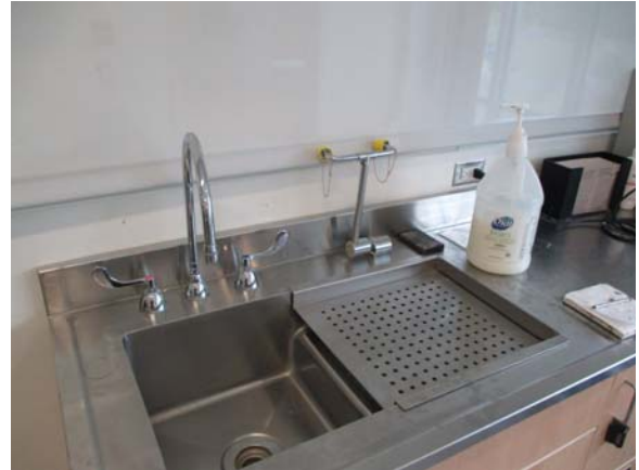
256083e 5/11/2021 Emergency eyewash adjacent to stainless steel lab sink Room 3207
