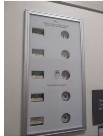
256094e 5/11/2021 Medical gas control valves for dental exam room Room 2103
