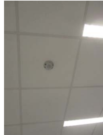
256082e 5/11/2021 Ceiling occupancy sensor Room 3207
