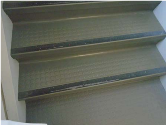
256091a 5/12/2021 Rubberized nosing and treads becoming worn Stairwell 2
