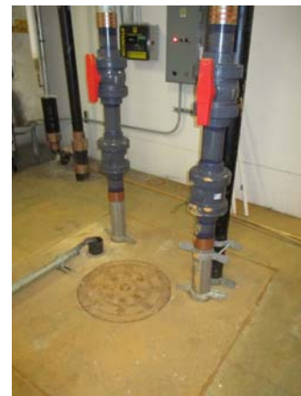
256120e 5/11/2021 Duplex sanitary lift station Room B0100
