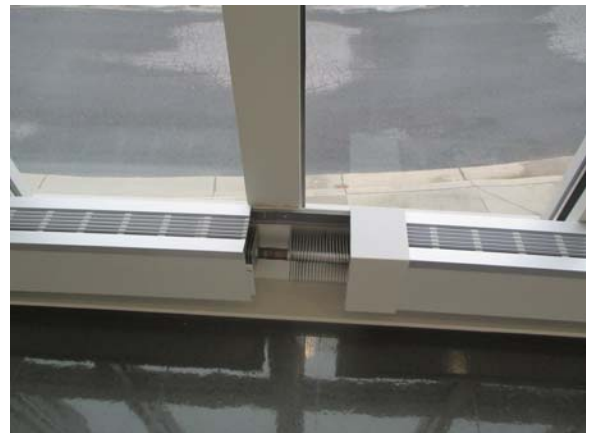
256087e 5/11/2021 Close-up of fin-tube radiator Third floor corridor
