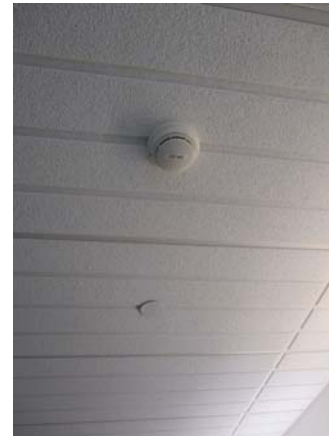
256080e 5/11/2021 Smoke/heat detector and recessed sprinkler head Third floor corridor
