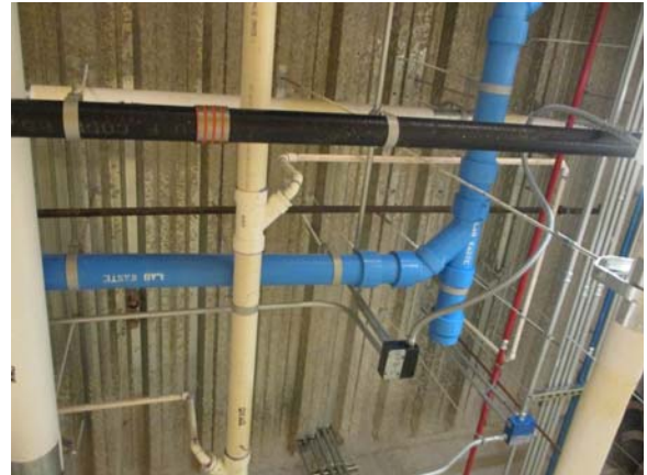
256125e 5/11/2021 Blue plastic lab waste drain piping Room B0100
