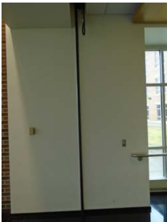
256105a 5/12/2021 Hidden fire screen Second floor by atrium
