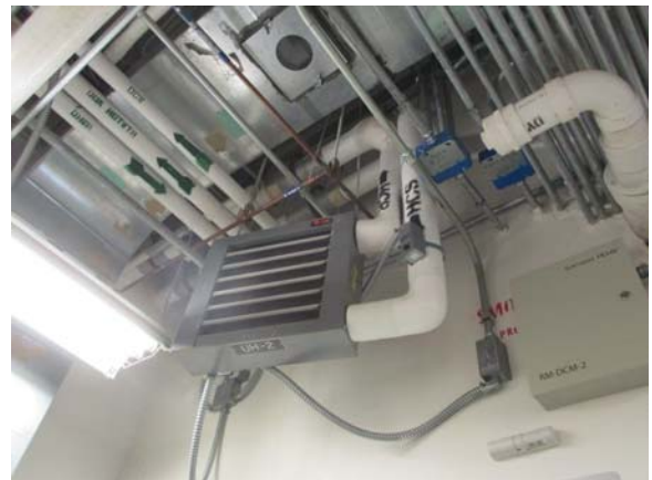
256102e 5/11/2021 One of two hot water unit heaters (UH-2) Loading dock
