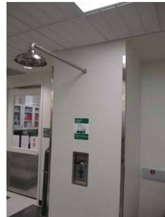
256069e 5/11/2021 Safety shower in large lab area Room 4200
