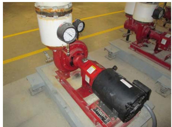
256051e 5/11/2021 Close-up of 10 hp HWP-1 Penthouse
