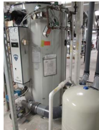
256045e 5/11/2021 Original 565 MBH PVI domestic water heater East end of penthouse
