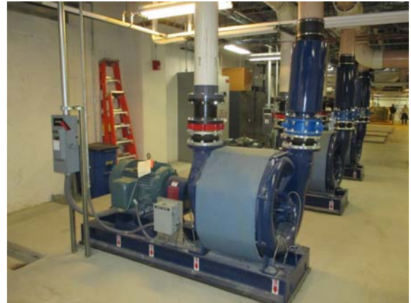
256112e 5/11/2021 Dental-mouth vacuum system with three 60 hp Spencer Turbines Room B0100
