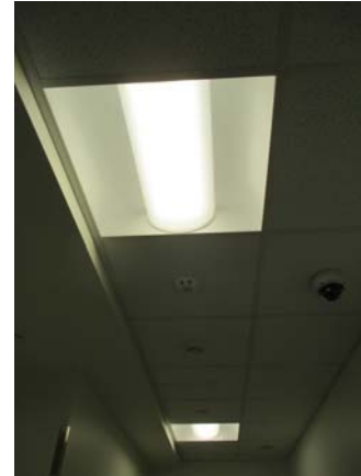
256056e 5/11/2021 Lay-in fluorescent light fixtures Fourth floor corridor
