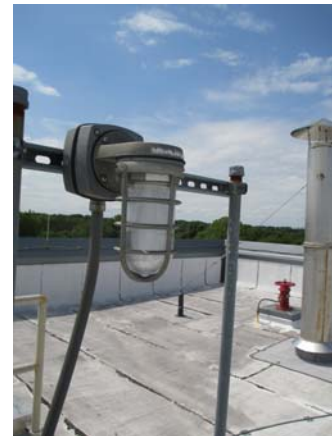
256011e 5/11/2021 CFL jelly-jar light fixture West end of roof
