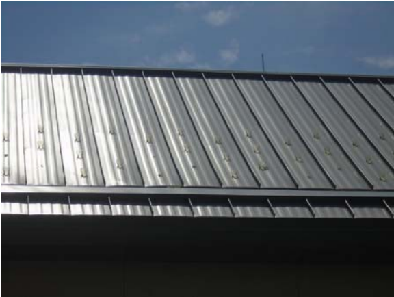
256028a 5/12/2021 Broken plastic "ice cleats" attached to metal roofing Pitched standing seam metal roof
