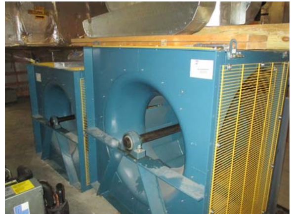
256032e 5/11/2021 Two original fans that were removed from AHU-L-1B because they were oversized Penthouse
