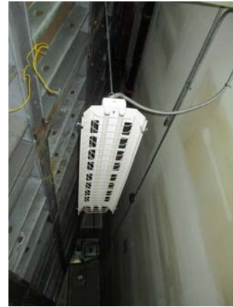
256019e 5/11/2021 Pendant fluorescent light fixture in mechanical space Top of atrium
