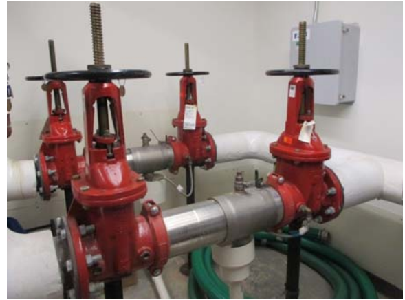
256107e 5/11/2021 Two 6 inch backflow preventers for domestic water Room 1259
