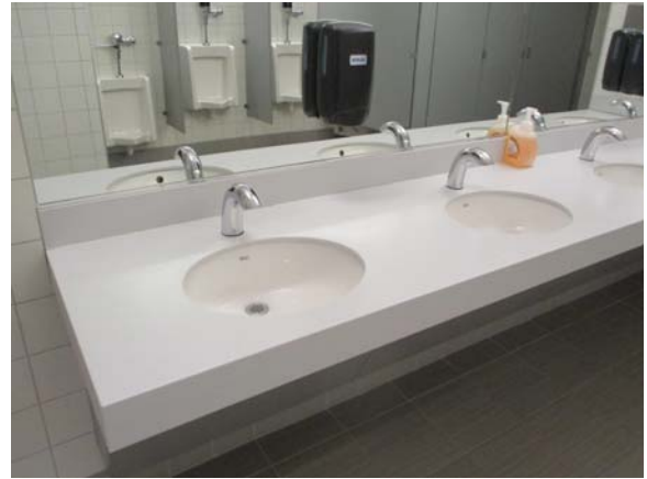
256077e 5/11/2021 Hands-free lavatories Fourth floor restroom
