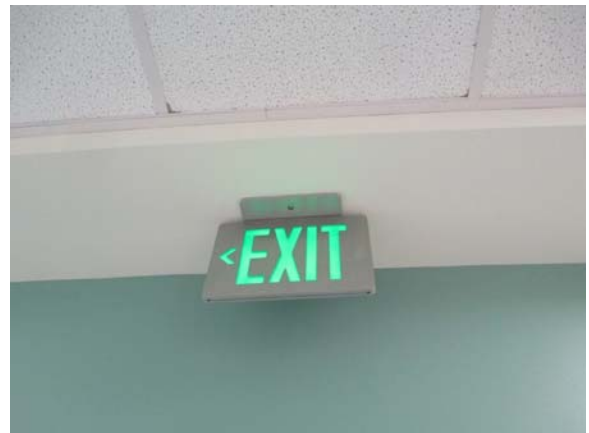
256057e 5/11/2021 LED exit sign Fourth floor corridor
