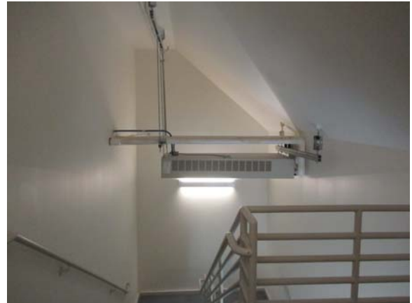
256028e 5/11/2021 Fan coil unit (FCU-5A1) at top of stairwell Top of stairwell S-1.5
