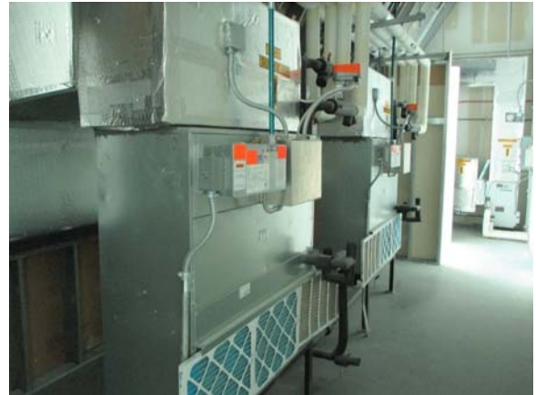
256017e 5/11/2021 Two Johnson Controls fan coil units Top of atrium
