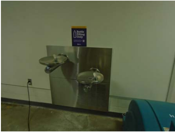
256122a 5/12/2021 Dual-level water fountain Basement
