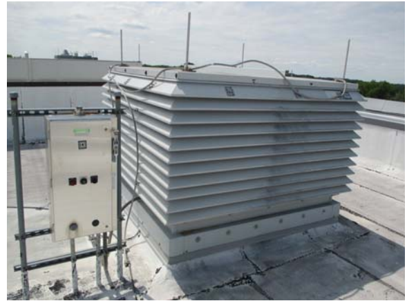
256013e 5/11/2021 Second 7.5 hp rectangular smoke exhaust fan (SF-E-2) Roof
