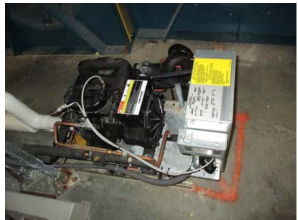
256033e 5/11/2021 Condensing unit for walk-in cold room Penthouse
