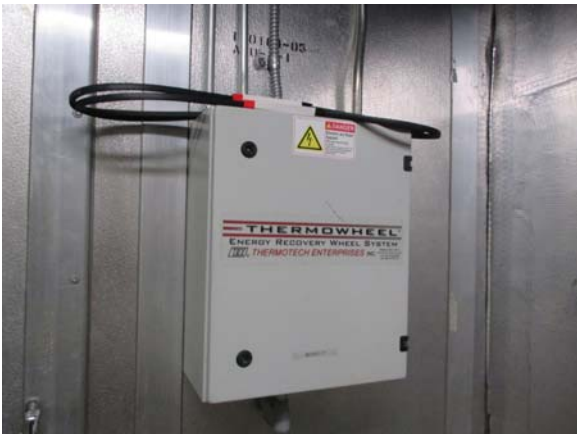
256130e 5/11/2021 Control box for the AHU-A-1 Thermotech Enterprises enthalpy wheel Room 3300
