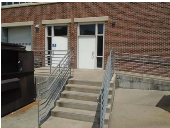
256015a 5/12/2021 Compliant ramp and handrailing for stepped entry West exterior
