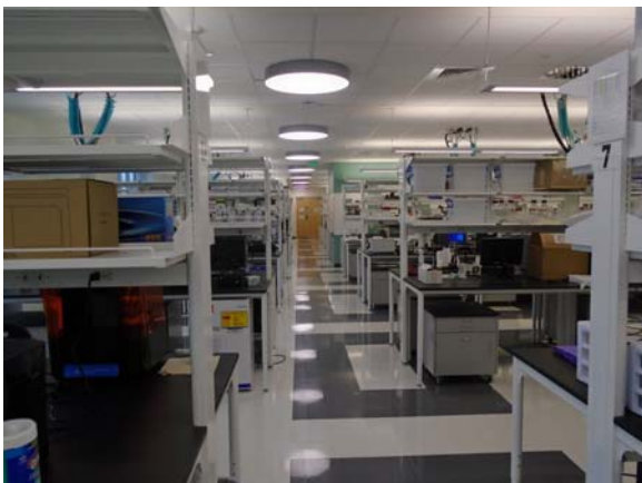
256048a 5/12/2021 Vinyl floor tile, suspended grid ceiling, and metal lab furniture Lab 4200
