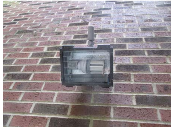
256007e 5/11/2021 Wall-mounted light fixture updated with LED bulb North exterior (stairwell)
