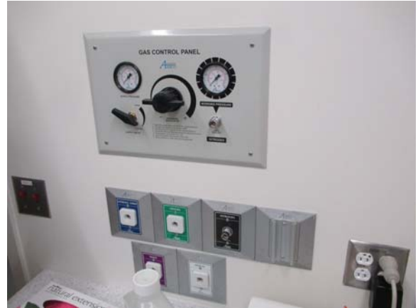
256095e 5/11/2021 Medical gas control panel for dental exam room Room 2103
