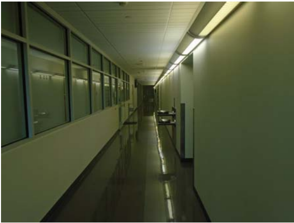
256077a 5/12/2021 Vinyl tile floor, painted walls, and suspended grid ceiling Third floor lab corridor
