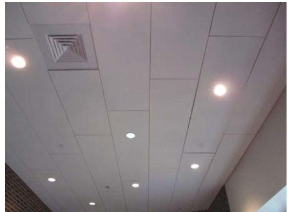
256096e 5/11/2021 Round recessed metal halide light fixtures outside lecture hall Lobby of lecture hall
