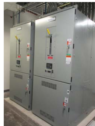
256099e 5/11/2021 Two Russelectric 1,000 amp ATS (LS and MEQ) Room E1180
