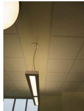
256066e 5/11/2021 Pendant LED light fixture in large lab area Room 4200
