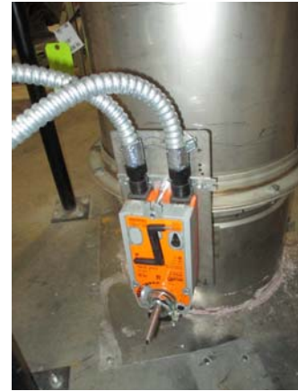
256026e 5/11/2021 Belimo electronic actuator on EX-L3 Northwest corner of penthouse
