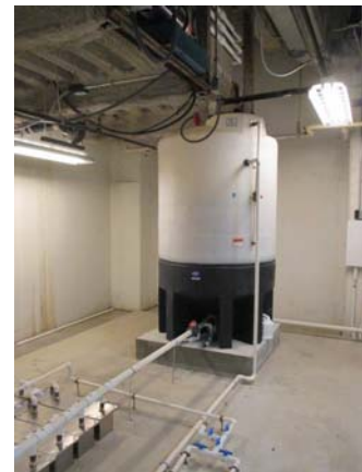
256111e 5/11/2021 Amalgam separator system Room B0100
