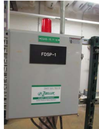
256118e 5/11/2021 Control panel for foundation sump pumps Room B0100
