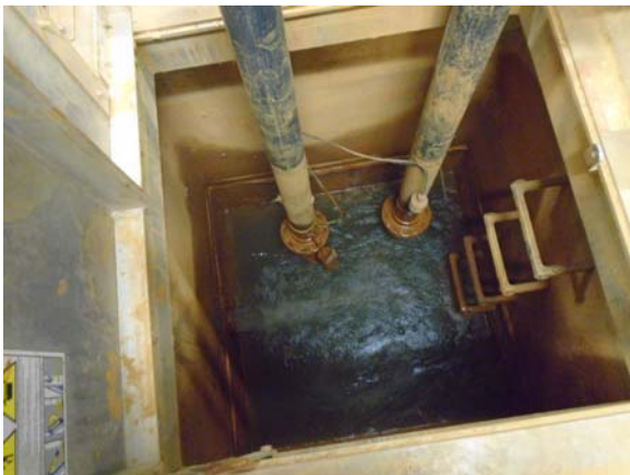
256123a 5/12/2021 Groundwater sump with two submerged pumps Basement
