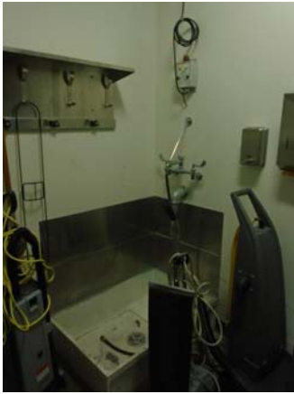
256121a 5/12/2021 Molded floor sink Basement janitorial closet
