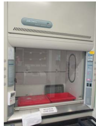
256084e 5/11/2021 Fume hood in lab area Room 3205
