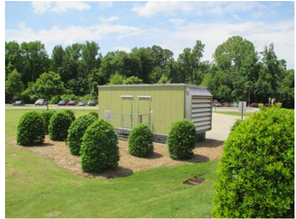
256004e 5/11/2021 750 kW emergency generator Southwest exterior
