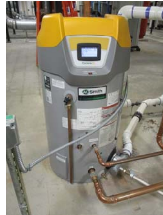
256044e 5/11/2021 Recently installed A. O. Smith domestic water heater East end of penthouse
