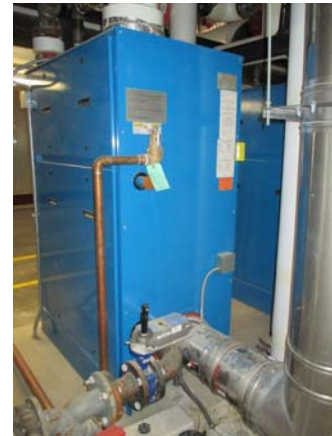
256041e 5/11/2021 One of four 2,500 MBH natural gas fired Harsco boilers (back side) East end of penthouse
