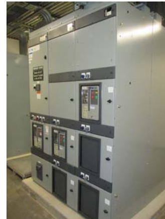
256098e 5/11/2021 1,600 amp switchgear for emergency generator Room E1180
