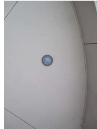
256002e 5/11/2021 Round recessed CFL light fixture North exterior at second floor entrance
