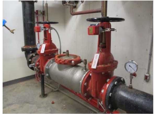
256106e 5/11/2021 8 inch backflow preventer for fire standpipe Room 1259
