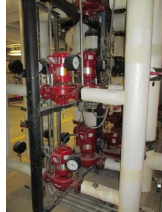
256050e 5/11/2021 Group of heating hot water pumps Penthouse
