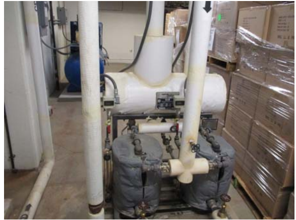
256127e 5/11/2021 Flash tank above condensate receiver Room B0100
