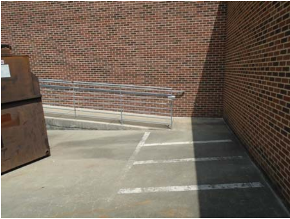
256016a 5/12/2021 Compliant ramp and handrailing for stepped entry West exterior
