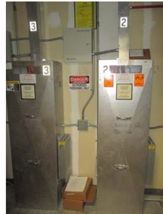
256074e 5/11/2021 Controls for the two passenger (traction) elevators Room 4105
