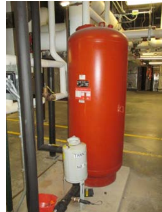
256043e 5/11/2021 Expansion tank (ET-1) for the heating hot water system East end of penthouse
