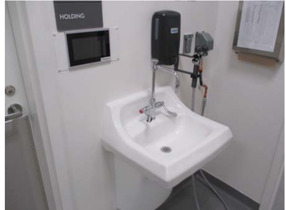
256059e 5/11/2021 Emergency eyewash mounted adjacent to wall-mounted lavatory Room 4210
