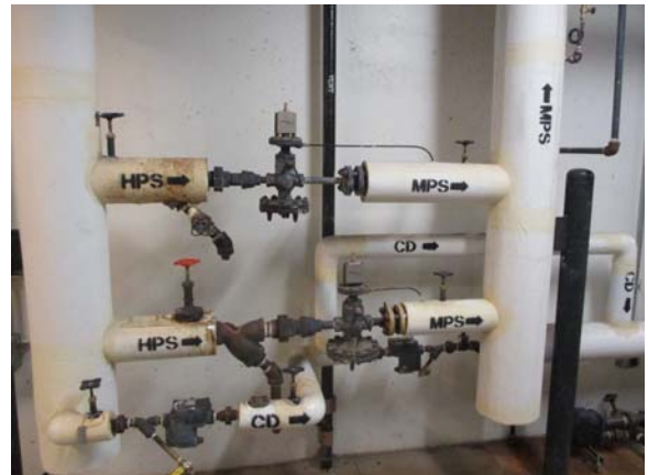
256126e 5/11/2021 Spirax Sarco pressure reducing valves Room B0100
