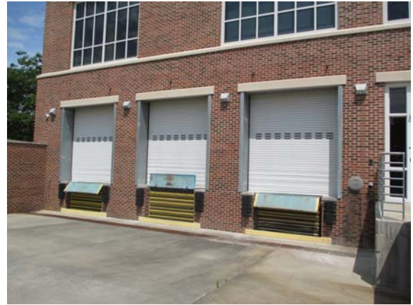
256005e 5/11/2021 Three dock levelers West loading docks
