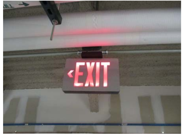
256022e 5/11/2021 Exit sign Northwest corner of penthouse
