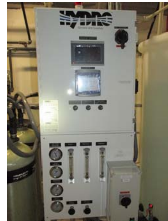
256040e 5/11/2021 Hydro control panel for RO/DI water system Southeast end of penthouse
