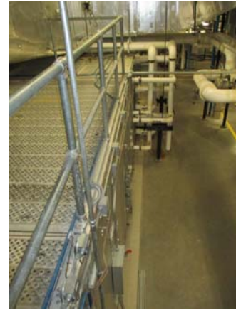
256038e 5/11/2021 A side of AHU-CL-2, with chilled water and heating hot water piping at far end Penthouse
