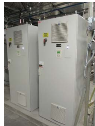
256030e 5/11/2021 Two VFDs for the supply fans (A and B) for AHU-CL-1 Penthouse
