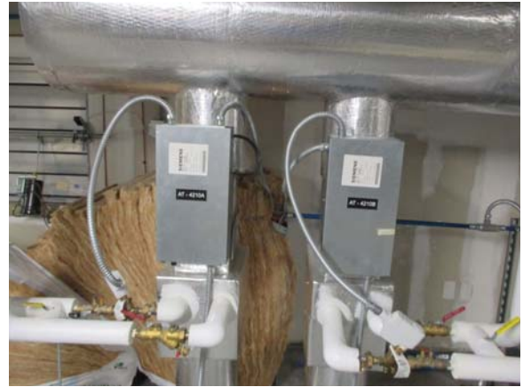
256020e 5/11/2021 Siemens controls on two hot water reheat coils in ductwork Northwest corner of penthouse
