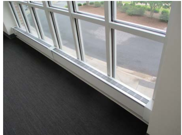
256086e 5/11/2021 Fin-tube radiators at base of windows Third floor corridor
