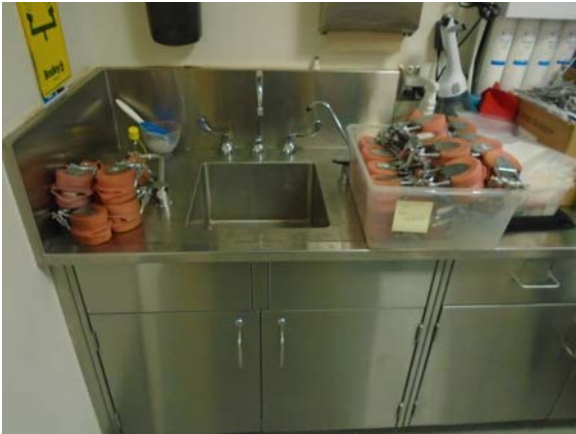
256082a 5/12/2021 Stainless steel lab sink Third floor labs
