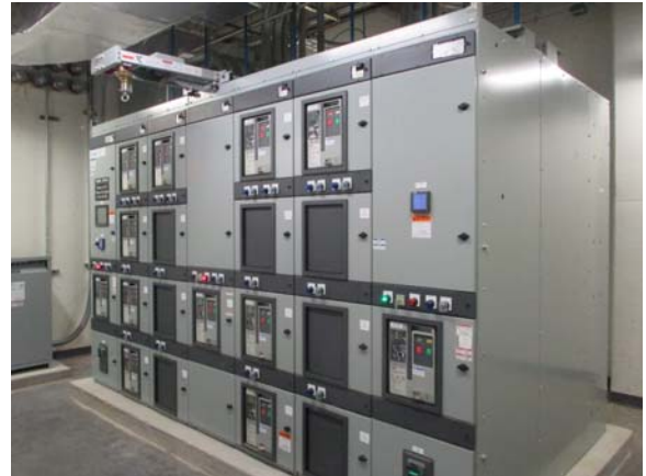
256100e 5/11/2021 Double-ended 3,200 amp main switchgear with tie-breaker Room E1182
