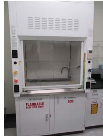
256064e 5/11/2021 Fume hood in lab area Room 4200
