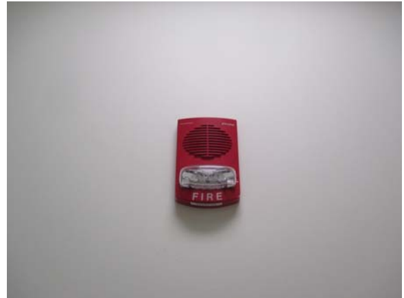
256058e 5/11/2021 Audible/visible fire device Fourth floor corridor
