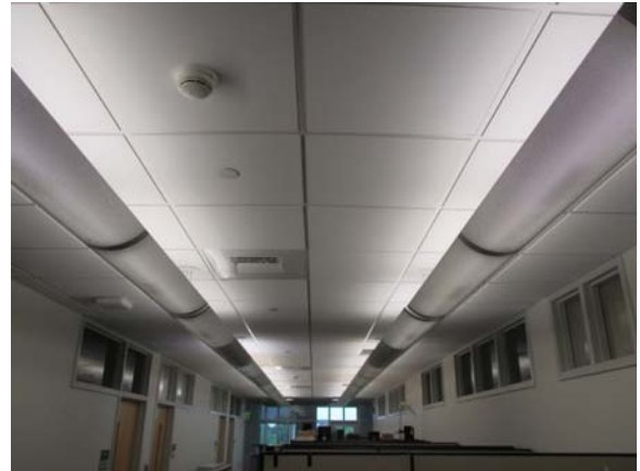
256088e 5/11/2021 Pendant fluorescent light fixtures above cubical office area Third floor corridor
