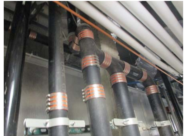
256035e 5/11/2021 No-hub cast-iron drain (vent) piping Penthouse
