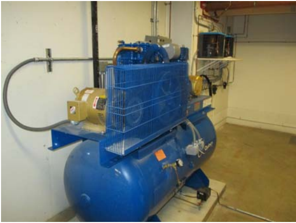
256128e 5/11/2021 Quincy air compressor with two 7.5 hp motors serving the HVAC controls Room B0100
