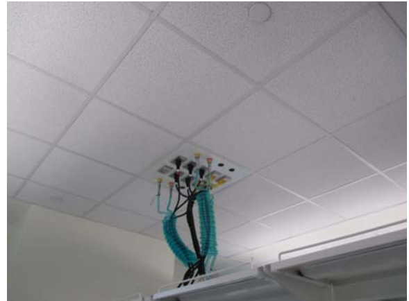
256067e 5/11/2021 Plumbing, power, and data connections enter the lab through the ceiling Room 4200
