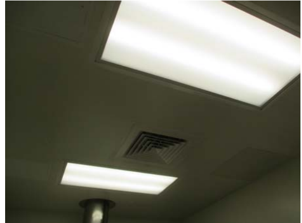
256062e 5/11/2021 2x4 lay-in LED light fixtures in lab area Room 4210C
