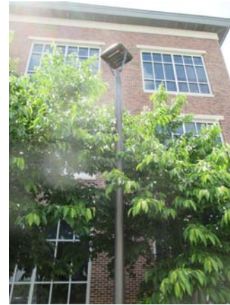
256001e 5/11/2021 LED light fixture on 15 foot stanchion Northwest exterior
