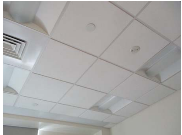
256085e 5/11/2021 Lay-in fluorescent light fixtures in office Room 3170
