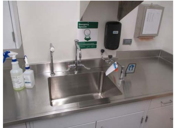
256061e 5/11/2021 Emergency eyewash adjacent to stainless steel lab sink Room 4210C
