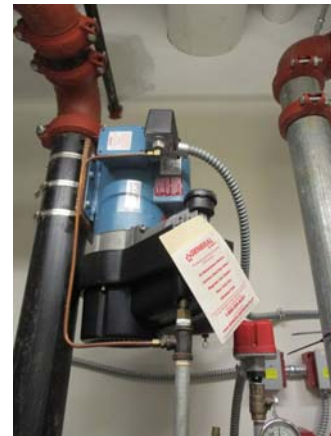
256108e 5/11/2021 Small air compressor for dry-pipe fire standpipe Room 1259
