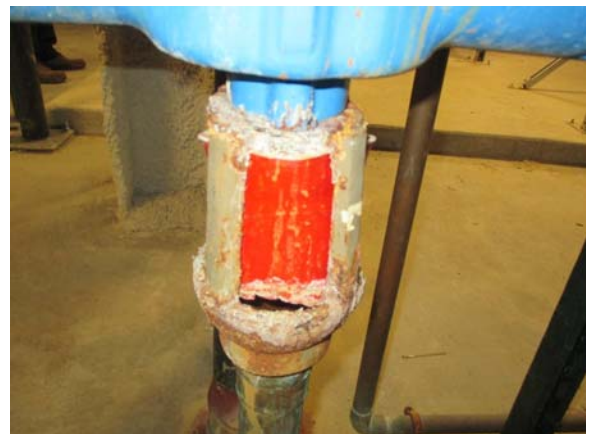
256048e 5/11/2021 Corrosion occurring at drain of backflow preventer East end of penthouse
