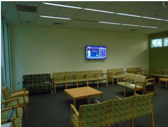
256110a 5/12/2021 Carpeting, painted walls, and suspended grid ceiling First floor waiting area
