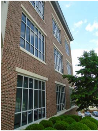
256004a 5/12/2021 Brick masonry exterior with cast concrete accents and dual-pane windows East exterior
