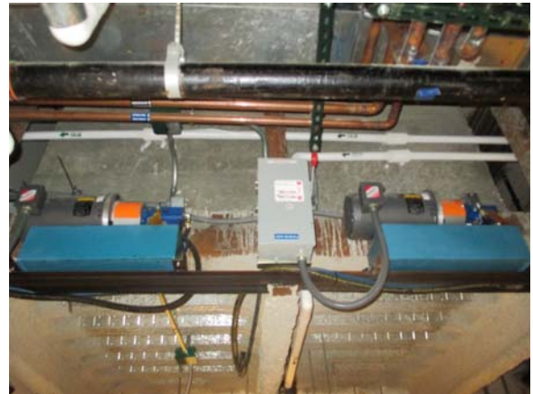
256110e 5/11/2021 Hydraulic pumps for two of the three dock levelers Room B0100
