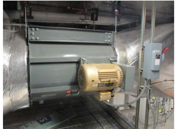
256031e 5/11/2021 One of two 25 hp return fans for AHU-CL-1 Penthouse
