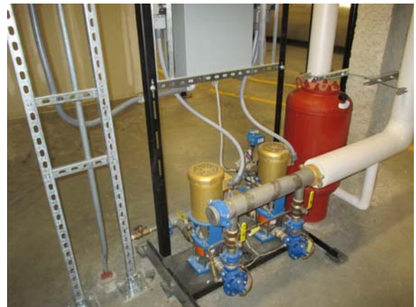
256054e 5/11/2021 Lab water booster pump system (PP1) Penthouse
