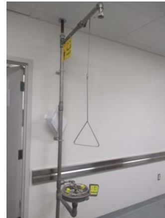
256104e 5/11/2021 Combination safety shower and eyewash station Room 1258
