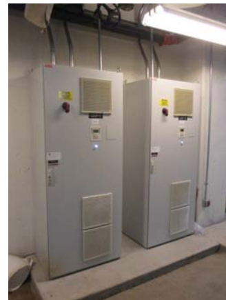
256123e 5/11/2021 VFDs for the two 40 hp chilled water pumps Room B0100
