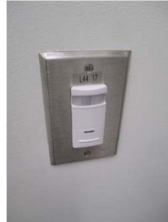
256065e 5/11/2021 Occupancy sensor built into light switch Alcove in room 4200
