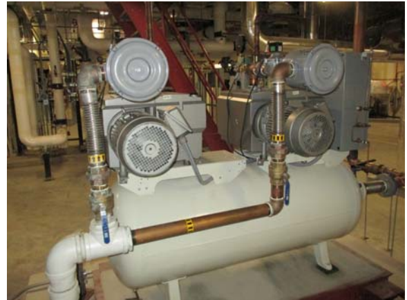
256049e 5/11/2021 Duplex vacuum system with two 5 hp motors Penthouse
