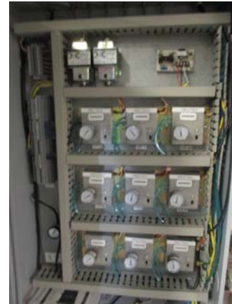
256052e 5/11/2021 Siemens control box for the pneumatic portion of HVAC controls Penthouse
