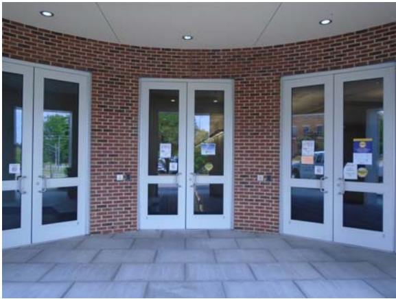
256002a 5/12/2021 Aluminum-framed glass entry doors with power openers Second floor east entry
