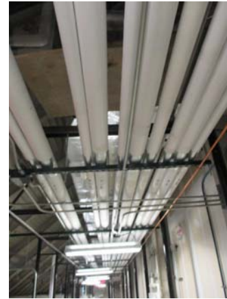
256034e 5/11/2021 Insulated piping running along the penthouse ceiling Penthouse
