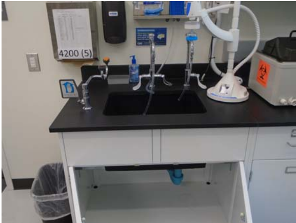
256049a 5/12/2021 Accessible lab sink Lab 4200
