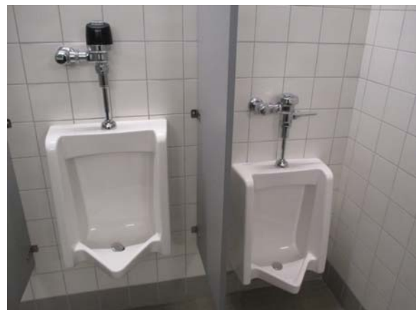
256078e 5/11/2021 Urinals in men's restroom Fourth floor restroom
