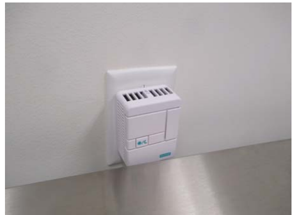
256063e 5/11/2021 Siemens thermostat for HVAC control Room 4210C
