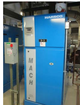
256042e 5/11/2021 Front side of Harsco B-3 boiler East end of penthouse
