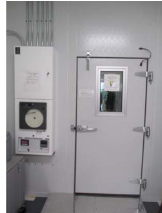
256068e 5/11/2021 Walk-in cold room South end of room 4200
