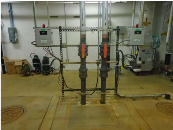
256125a 5/12/2021 Groundwater sump with two submerged pumps Basement
