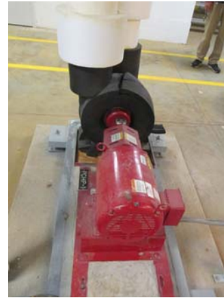
256121e 5/11/2021 7.5 hp PCHP-1 chilled water pump Room B0100
