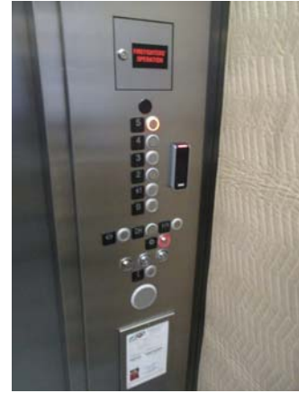
256008e 5/11/2021 Control panel for freight elevator Freight elevator interior
