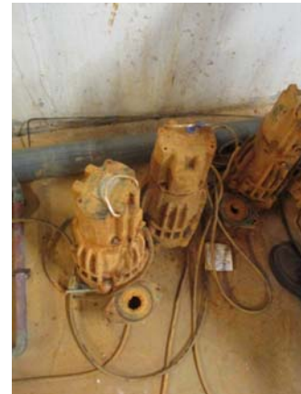
256116e 5/11/2021 Failed sump pumps, clogged with mud Room B0100
