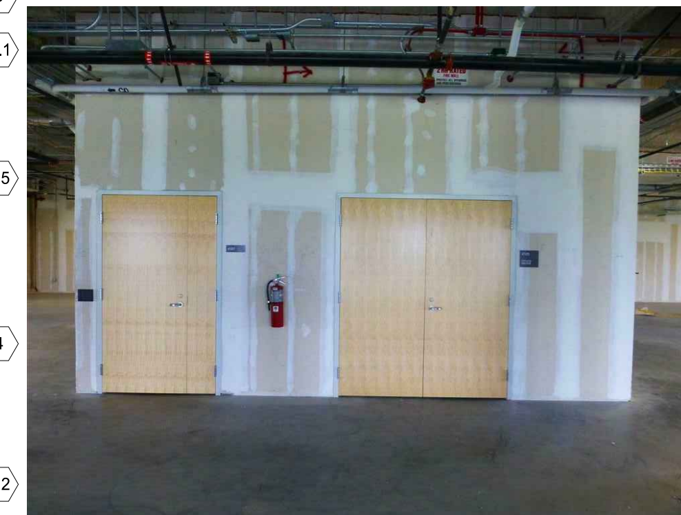
IMAGE C: EXISTING WALLS AT INTERIOR ONE CARD AND ELEV/MACH ROOM. INTERIOR WALL BETWEEN ATRIUM AND SHELL SPACE VISIBLE BEYOND.
