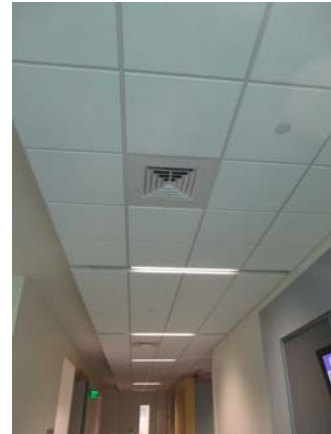
256070e 5/11/2021 T5 fluorescent light fixtures in the elevator lobby Fourth floor corridor
