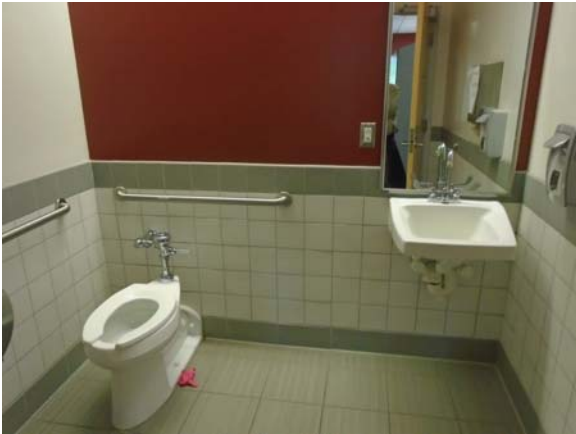
256095a 5/12/2021 Ceramic tile floor and lower wall, painted wall above, accessible fixtures Unisex restroom
