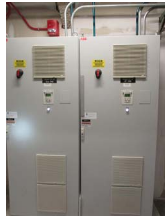
256036e 5/11/2021 VFDs for both the supply and return fans (A and B side) of AHU-CL-2 Penthouse
