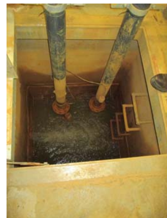
256117e 5/11/2021 Pit with two sump pumps for problematic foundation infiltration Room B0100
