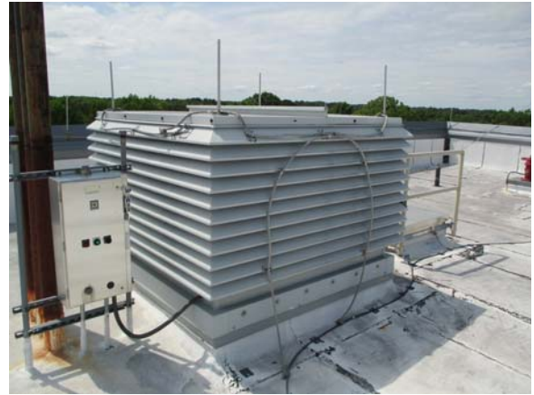
256010e 5/11/2021 7.5 hp rectangular fan (SF-E-1) provides elevator pressurization West end of roof
