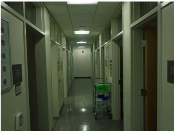
256113a 5/12/2021 Vinyl tile floor, painted walls, and suspended grid ceiling First floor lab corridor
