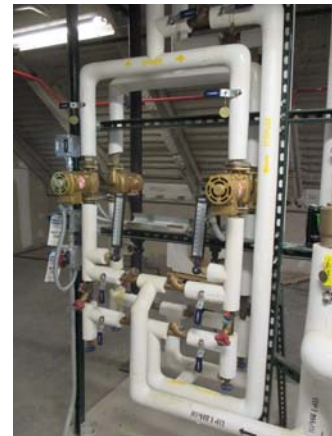
256046e 5/11/2021 Four fractional horsepower pumps for various water piping East end of penthouse
