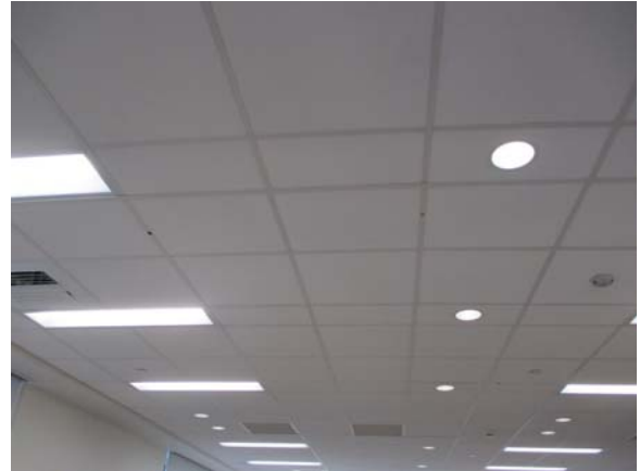
256092e 5/11/2021 Lay-in fluorescent light fixtures in large dental chair area Room 2010
