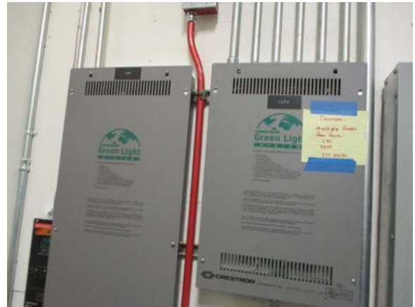
256071e 5/11/2021 Creston lighting control panels Room 4101
