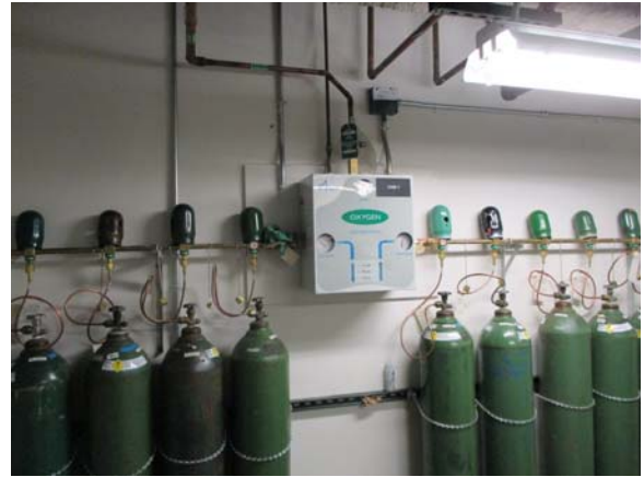
256109e 5/11/2021 Oxygen gas manifold Room B0101
