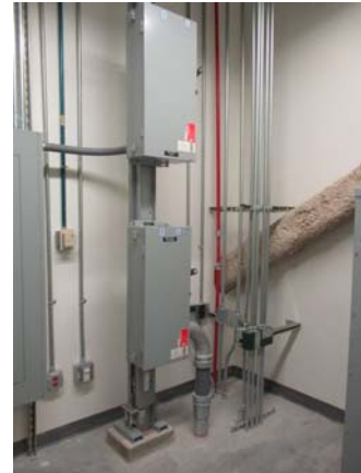
256073e 5/11/2021 480 volt electrical bus duct Room 4101A
