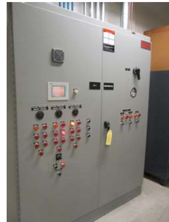
256113e 5/11/2021 Control panel for Spencer Turbines Room B0100
