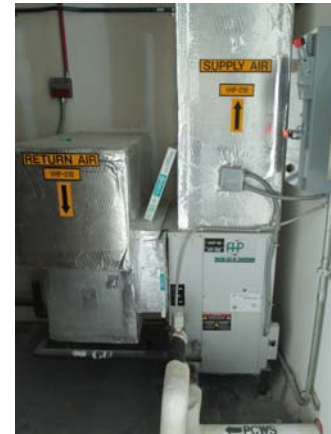
256018e 5/11/2021 FHP heat pump (HP-5B1) Top of atrium
