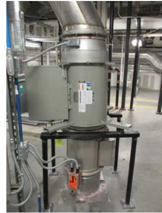
256025e 5/11/2021 Axial/mixed-flow fan (EX-L3) Northwest corner of penthouse
