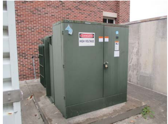
256055e 5/11/2021 2,000 KVA oil-filled transformer Southeast exterior
