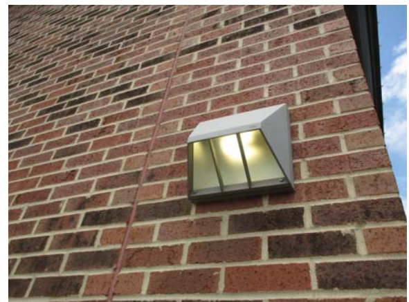
256003e 5/11/2021 Wall-mounted CFL light fixture West exterior
