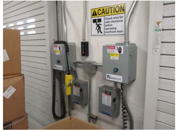
256103e 5/11/2021 Hydraulic dock leveler controls Loading dock
