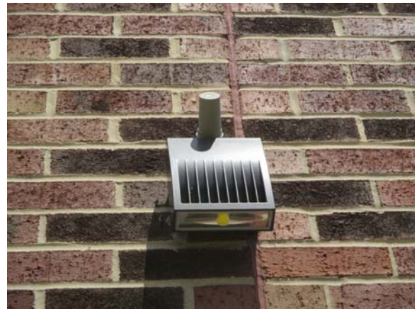
256006e 5/11/2021 Wall-mounted LED light fixture West exterior
