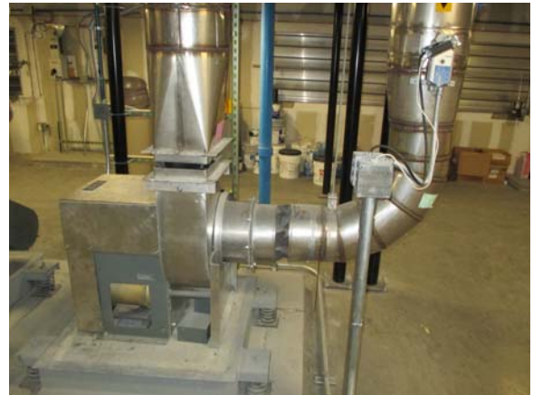
256023e 5/11/2021 1 hp exhaust fan (EX-16) Northwest corner of penthouse
