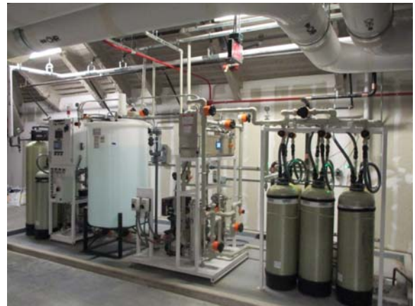
256039e 5/11/2021 RO/DI water system supplying DI water to the labs Southeast end of penthouse
