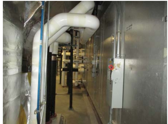
256029e 5/11/2021 Large air handling unit (AHU-CL-1) with chilled water and heating hot water piping at far end Penthouse
