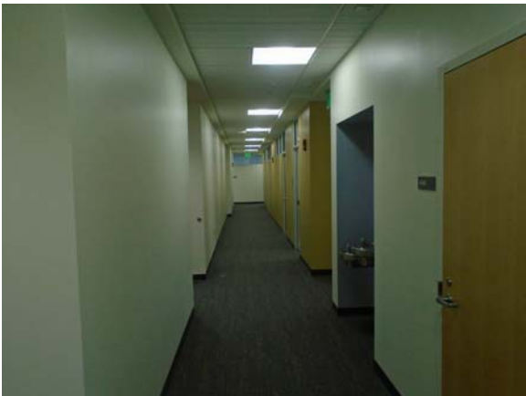
256060a 5/12/2021 Carpeting, painted walls, and suspended grid ceiling Fourth floor office suite corridor
