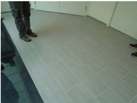
256057a 5/12/2021 Ceramic tile floor adjacent to a terrazzo floor Fourth floor balcony area
