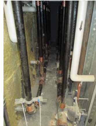
256076e 5/11/2021 Insulated supply piping and cast-iron drain piping Pipe chase behind fourth floor restrooms
