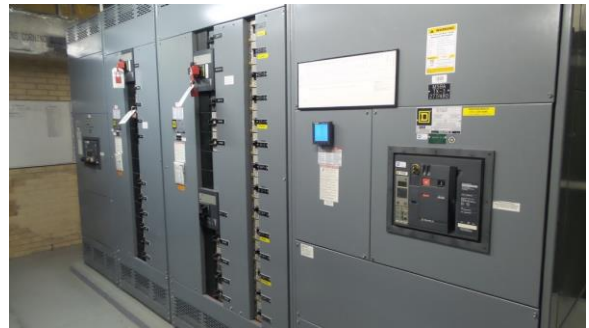
HSCW040e 4/18/2016 Low-voltage switchgear MSBA CUP, room 133
