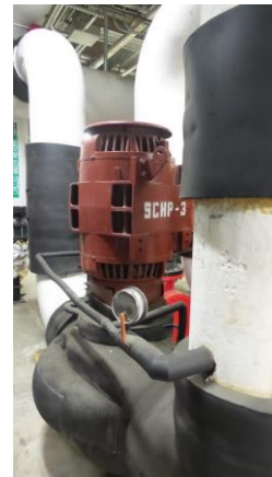
HSCW010e 4/18/2016 5,000 GPM pump SCHP-3 with 100 hp motor CUP, first floor
