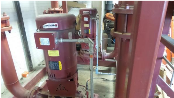
HSCW027e 4/18/2016 Booster pumps with 15 hp motors CUP, first floor
