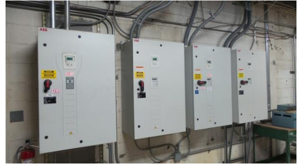
HSCW002e 4/18/2016 Variable frequency drives for chilled water pumps CUP, first floor
