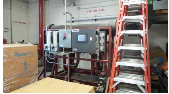
HSCW026e 4/18/2016 Booster pump control equipment CUP, first floor
