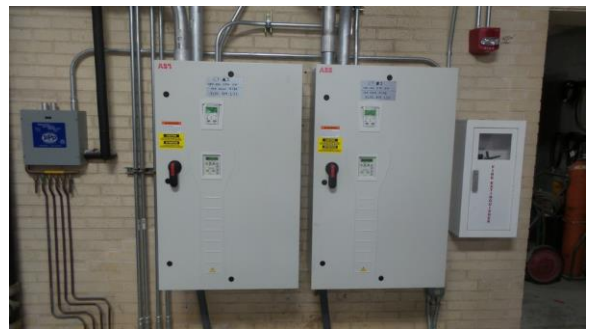
HSCW042e 4/18/2016 Variable frequency drives for cooling tower fans CUP, first floor
