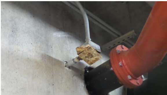
HSCW069e 4/18/2016 Corroded junction box Utility tunnel extension 850 foot
