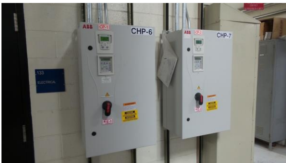
HSCW029e 4/18/2016 Variable frequency drives for chilled water pumps CUP, first floor
