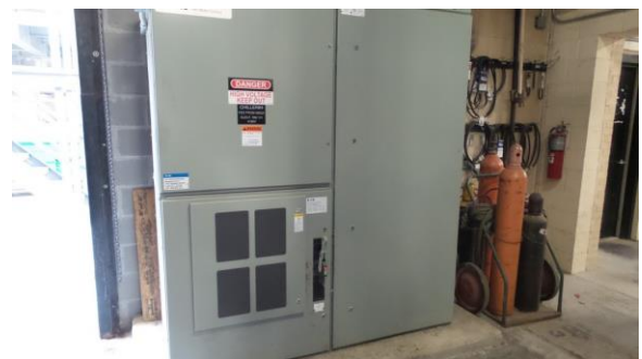
HSCW018e 4/18/2016 CH-4 motor starter rated for 5 kV CUP, first floor
