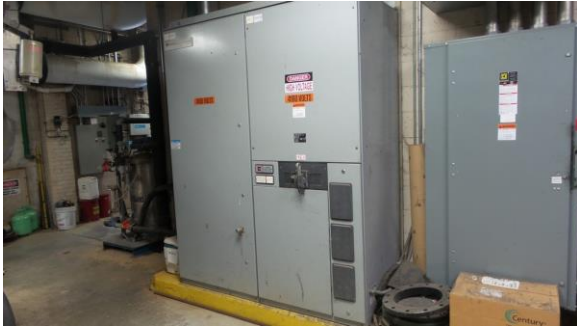
HSCW013e 4/18/2016 CH-3 motor starter rated for 5 kV CUP, first floor
