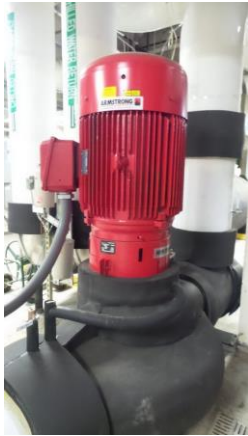
HSCW007e 4/18/2016 5,000 GPM pump SCHP-1 with 100 hp motor CUP, first floor
