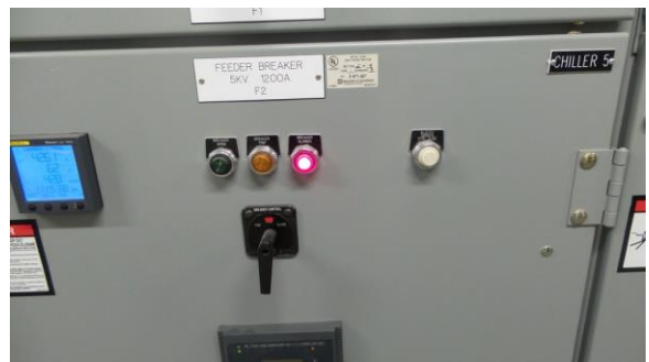
HSCW036e 4/18/2016 Vacuum breaker for Chiller 5 CUP, room 131
