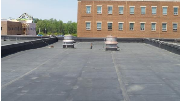
HSCW049e 4/18/2016 Rooftop exhaust fans CUP roof
