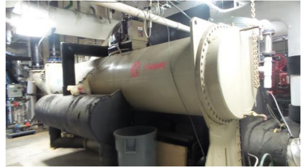
HSCW008e 4/18/2016 Trane centrifugal water-cooled chiller CH-3 rated for 1,000 tons CUP, first floor
