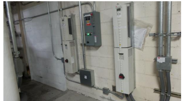
HSCW004e 4/18/2016 Variable frequency drives for chilled water pumps CUP, first floor
