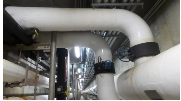
HSCW068e 4/18/2016 Chilled water supply and return to Dental Utility tunnel extension
