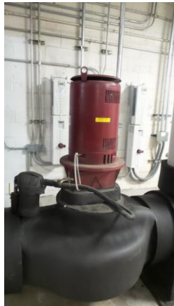
HSCW003e 4/18/2016 2,000 GPM pump CHP-7 with 25 hp motor CUP, first floor
