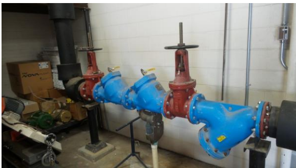
HSCW023e 4/18/2016 6 inch domestic water backflow preventer CUP, first floor
