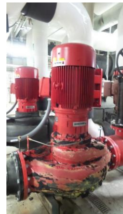
HSCW006e 4/18/2016 5,000 GPM pump SCHP-4 with 100 hp motor CUP, first floor
