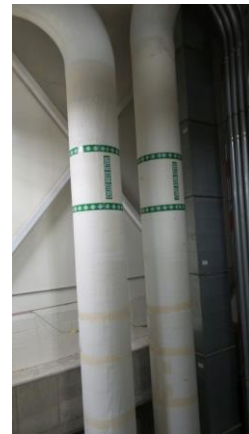
HSCW034e 4/18/2016 Chilled water supply and return pipe CUP, first floor
