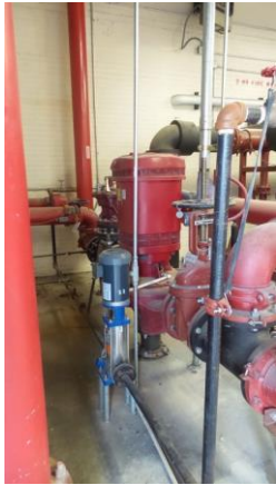
HSCW025e 4/18/2016 Fire pump and associated jockey pump CUP, first floor
