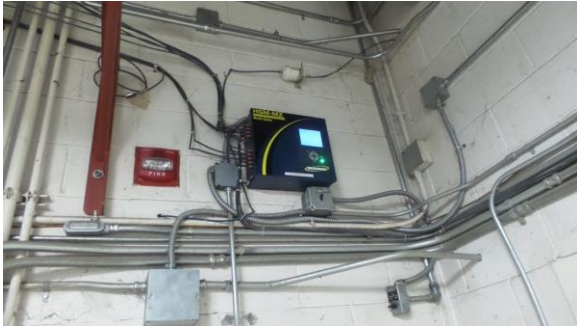
HSCW001e 4/18/2016 Refrigerant monitoring system CUP, first floor
