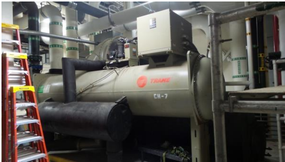
HSCW033e 4/18/2016 Trane centrifugal water-cooled chiller CH-7 rated for 1,000 ton CUP, first floor
