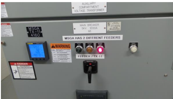
HSCW035e 4/18/2016 Vacuum breaker cabinet MSGA TX-11 CUP, room 131
