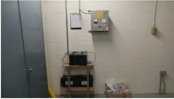
HSCW037e 4/18/2016 Battery charger and battery bank CUP, room 131
