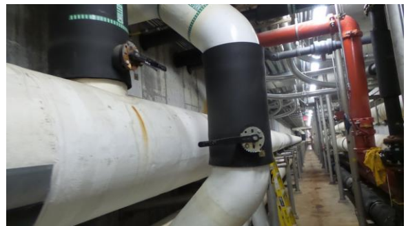
HSCW060e 4/18/2016 Isolation valves Original utility tunnel
