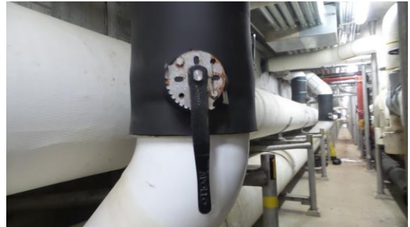
HSCW058e 4/18/2016 Isolation valve Original utility tunnel
