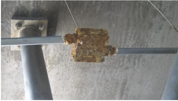
HSCW067e 4/18/2016 Corroded junction box Utility tunnel extension 800 foot
