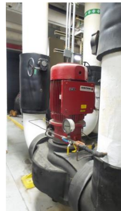
HSCW030e 4/18/2016 2,400 GPM pump CHP-6 with 40 hp motor CUP, first floor
