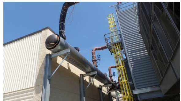
HSCW048e 4/18/2016 Condenser water common header CUP exterior
