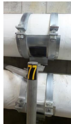
HSCW066e 4/18/2016 Pipe guide, anchor, stanchion and saddle Utility tunnel extension 770 foot
