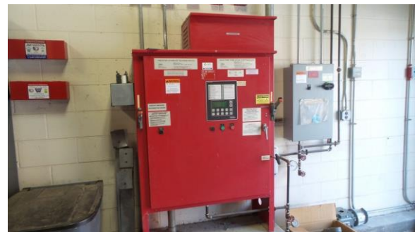
HSCW024e 4/18/2016 Fire pump controller CUP, first floor
