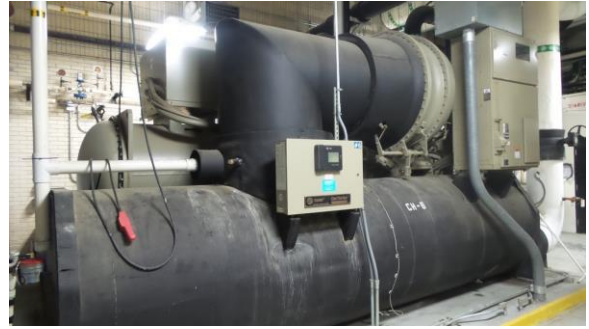
HSCW032e 4/18/2016 Trane centrifugal water-cooled chiller CH-6 rated for 1,000 ton CUP, first floor
