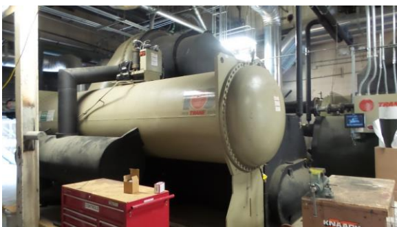
HSCW017e 4/18/2016 Trane centrifugal water-cooled chiller CH-4 rated for 1,400 tons CUP, first floor
