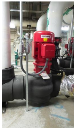
HSCW005e 4/18/2016 2,400 GPM pump CHP-3 with 40 hp motor CUP, first floor
