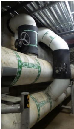
HSCW053e 4/18/2016 Chilled water pipe, valves and support equipment Original utility tunnel
