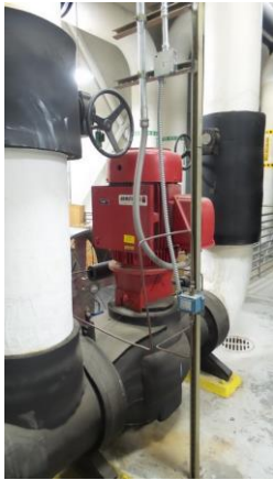
HSCW031e 4/18/2016 2,400 GPM pump CHP-7 with 40 hp motor CUP, first floor
