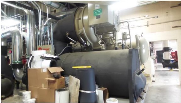
HSCW021e 4/18/2016 Trane centrifugal water-cooled chiller CH-5 rated for 1,400 tons CUP, first floor
