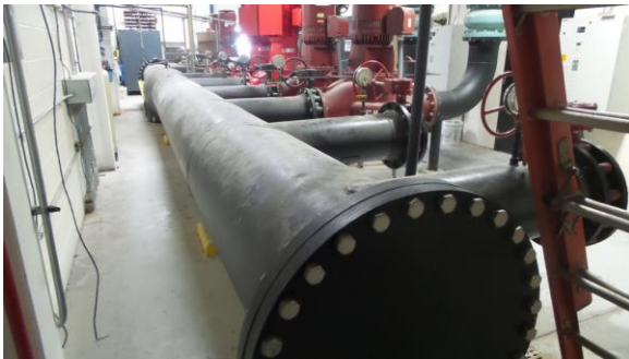
HSCW045e 4/18/2016 Condenser water common header CUP, first floor
