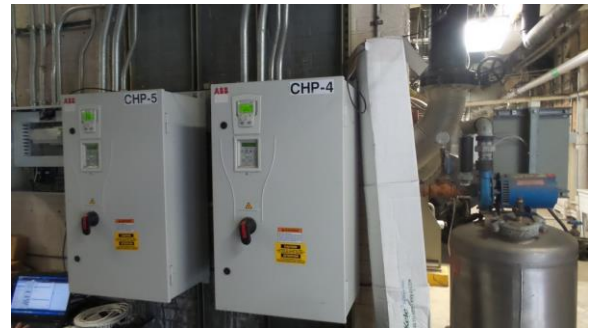
HSCW016e 4/18/2016 Variable frequency drives for chilled water pumps CUP, first floor
