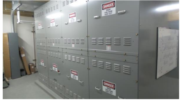
HSCW038e 4/18/2016 Rear access to switchgear MSGA CUP, room 131
