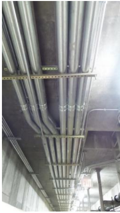
HSCW061e 4/18/2016 High voltage conduit Original utility tunnel
