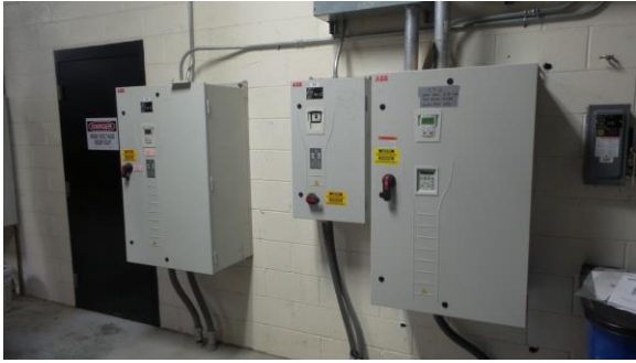
HSCW043e 4/18/2016 Variable frequency drives for pumps and cooling tower fan CUP, first floor
