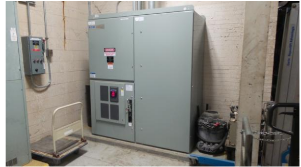
HSCW022e 4/18/2016 CH-5 motor starter rated for 5 kV CUP, first floor
