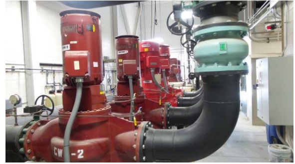
HSCW044e 4/18/2016 Six condenser water pumps CUP, first floor
