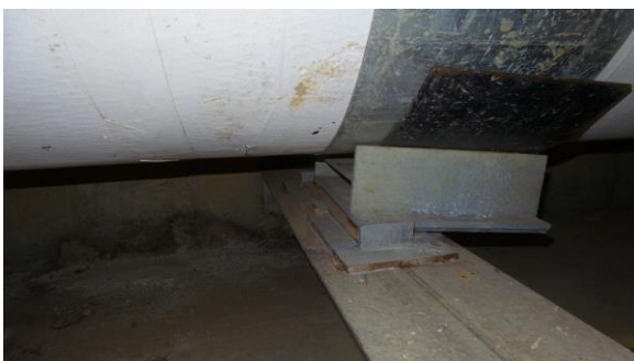
HSCW065e 4/18/2016 Evidence of pipe movement Utility tunnel extension 630 foot
