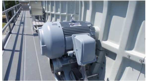
HSCW052e 4/18/2016 Cooling tower fan motor CUP roof
