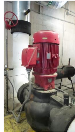
HSCW020e 4/18/2016 2,400 GPM pump CHP-5 with 40 hp motor CUP, first floor
