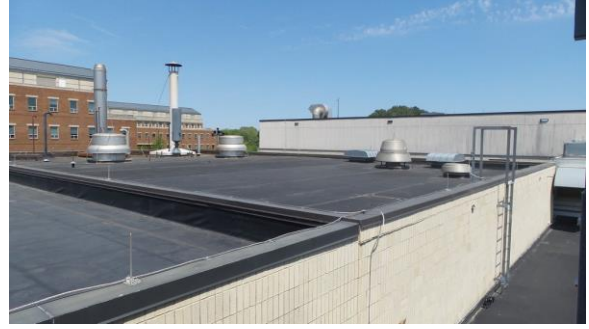
HSCW050e 4/18/2016 Rooftop exhaust fans CUP roof
