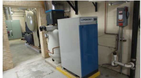
HSCW028e 4/18/2016 Air compressor, air dryer and air storage tank CUP, first floor
