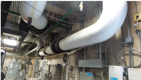
HSCW015e 4/18/2016 Chilled water system crossover bridge CUP, first floor
