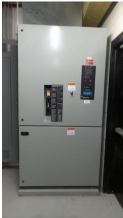
HSCW039e 4/18/2016 Automatic transfer switch ATS-EQ CUP, room 133
