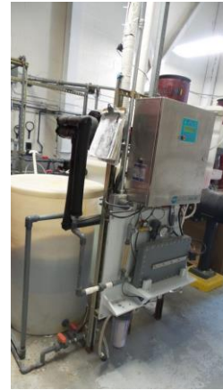
HSCW046e 4/18/2016 Cooling tower and condenser water treatment equipment CUP, first floor
