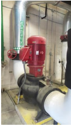
HSCW019e 4/18/2016 2,400 GPM pump CHP-4 with 40 hp motor CUP, first floor
