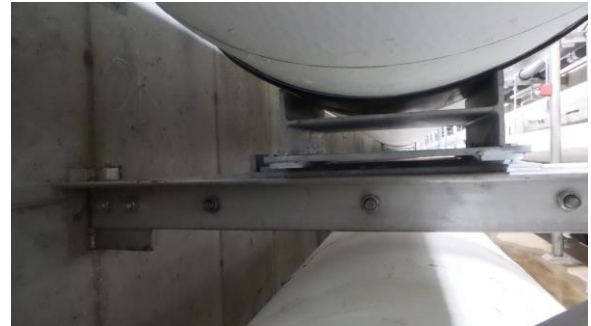
HSCW064e 4/18/2016 Pipe saddle and wall anchor Utility tunnel extension
