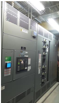
HSCW041e 4/18/2016 Low-voltage switchgear MSBB CUP, room 133
