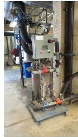
HSCW014e 4/18/2016 Sand filter system CUP, first floor
