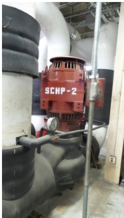
HSCW009e 4/18/2016 5,000 GPM pump SCHP-2 with 100 hp motor CUP, first floor
