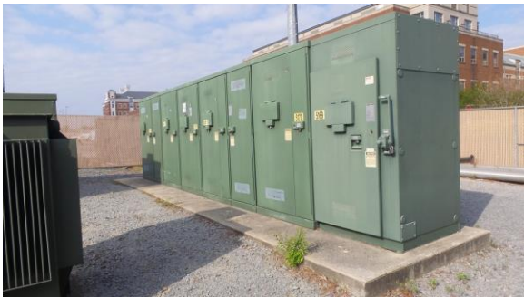
HSEL015e 4/21/2016 Utility system load interrupter switches Main substation
