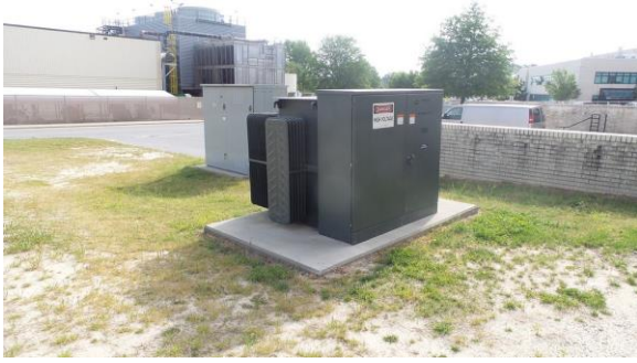
HSEL025e 4/21/2016 Transformer TX-10A Warren Life Sciences exterior
