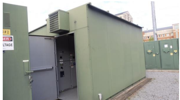
HSEL004e 4/21/2016 Electrical GUC POD #1 Main substation
