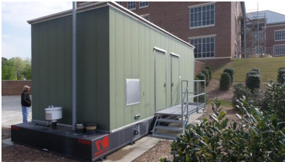
HSEL033e 4/21/2016 750 kW emergency generator building Ross Hall exterior
