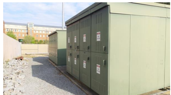
HSEL012e 4/21/2016 Exterior bus access to POD #1 and POD #2 Main substation
