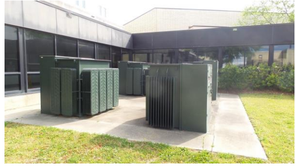
HSEL038e 4/21/2016 Four oil-filled transformers Brody exterior
