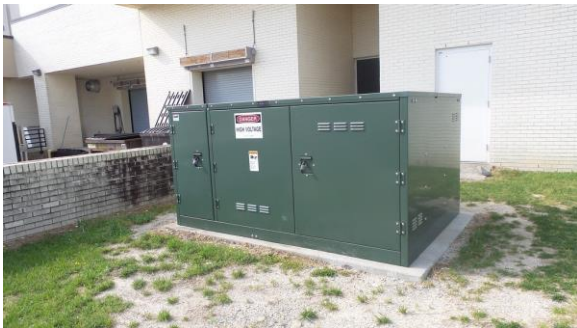
HSEL021e 4/21/2016 Five-way switch HVSS7 Warren Life Sciences exterior
