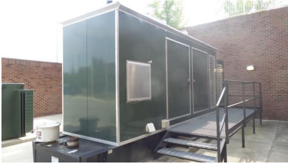
HSEL037e 4/21/2016 250 kW emergency generator housing Family Medicine exterior
