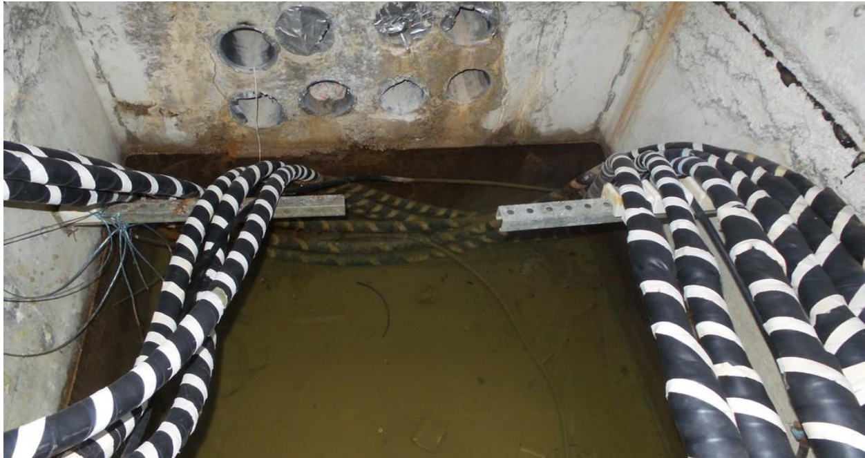
Image 3: 15 kV cable submerged in standing water within a utility vault
