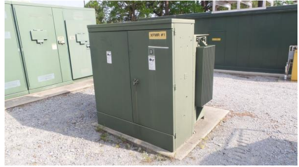
HSEL014e 4/21/2016 Oil-filled transformer #1 Main substation
