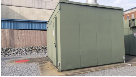
HSEL001e 4/21/2016 Electrical GUC POD #2 Main substation
