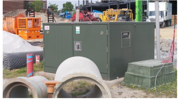
HSEL026e 4/21/2016 Selector switch HVSS8 New Student Union exterior
