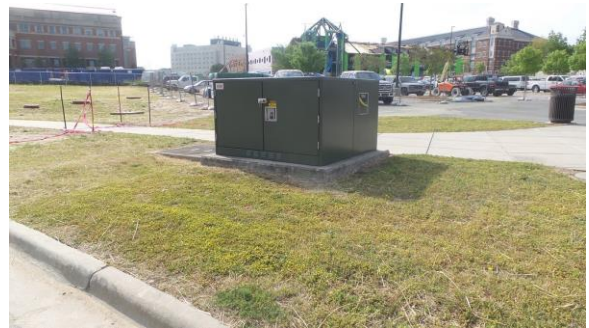
HSEL034e 4/21/2016 Selector switch HVSS10 Between Allied and Ross
