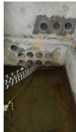
HSEL042e 4/21/2016 Standing water in manhole Between Brody and Life Sciences
