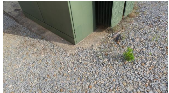
HSEL010e 4/21/2016 Concrete transformer pad Main substation
