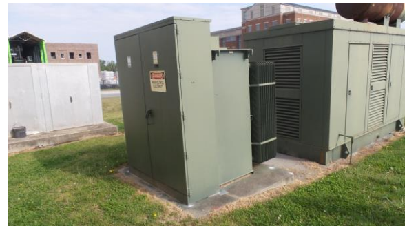
HSEL022e 4/21/2016 Transformer TX-10 Warren Life Sciences exterior
