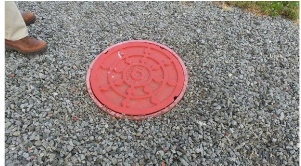
HSEL040e 4/21/2016 Electrical vault/manhole cover Between Brody and Life Sciences
