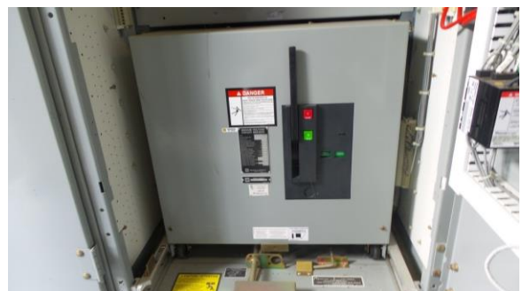
HSEL006e 4/21/2016 1,200 amp vacuum circuit breaker GUC POD #1
