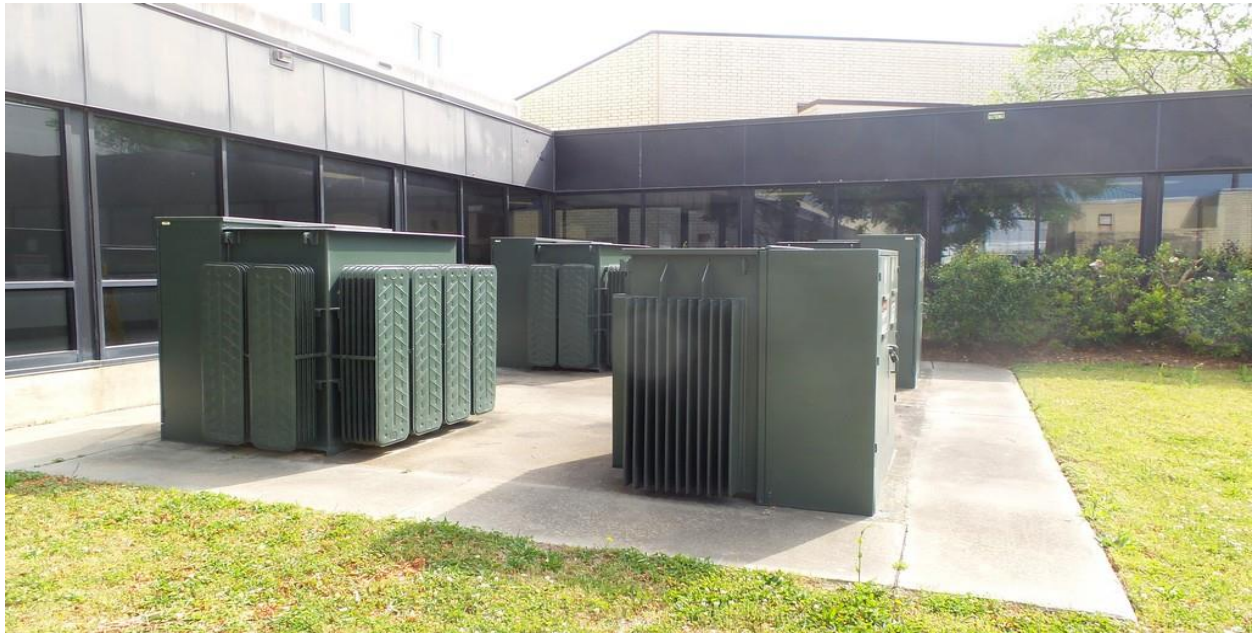
Image 2: Transformers TX-4, TX-5, TX-6, and TX-7 at Brody
