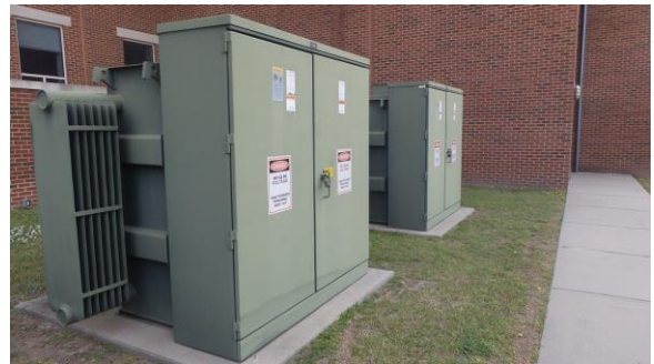
HSEL028e 4/21/2016 Transformers TX15 and TX16 Allied Health exterior
