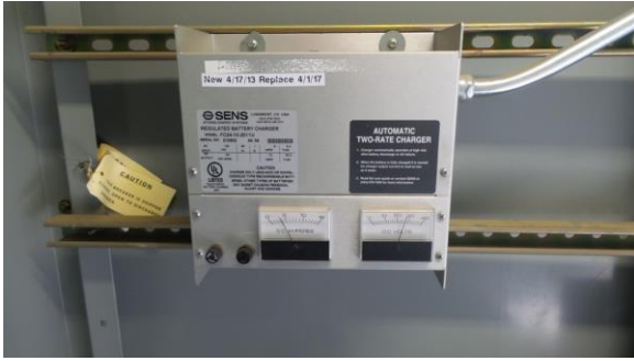
HSEL007e 4/21/2016 Battery charger GUC POD #1
