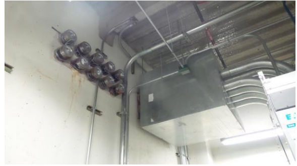
HSEL032e 4/21/2016 Installed conduit for second transformer and feeder circuit Ross Hall, room 1182
