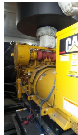
HSEL018e 4/21/2016 1,250 kW CUP emergency generator Main substation
