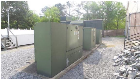
HSEL009e 4/21/2016 Selector switch HVSS3 and transformers Main substation
