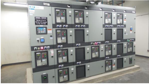
HSEL031e 4/21/2016 3,000 amp, 480 volt normal service switchgear Ross Hall, room 1182
