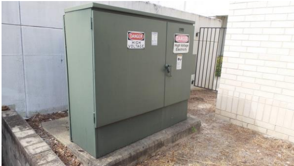
HSEL039e 4/21/2016 Oil-filled transformer TX-9 Biotech exterior
