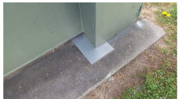
HSEL024e 4/21/2016 Damaged and repaired concrete slab Warren Life Sciences exterior
