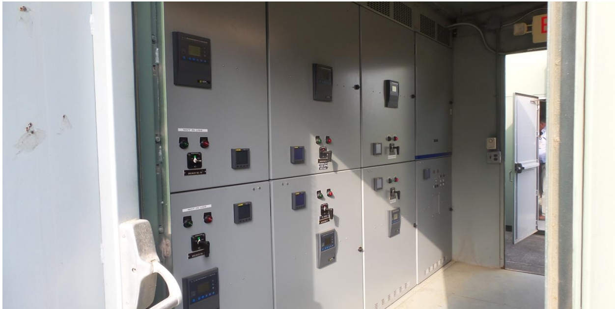
Image 1: Metalclad Switchgear MSG2
