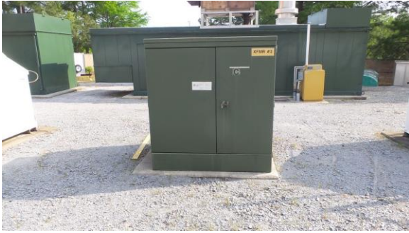
HSEL013e 4/21/2016 Oil-filled transformer #2 Main substation
