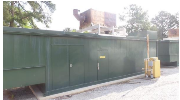
HSEL016e 4/21/2016 Utility system emergency generator building Main substation
