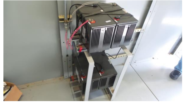
HSEL008e 4/21/2016 Battery bank GUC POD #1
