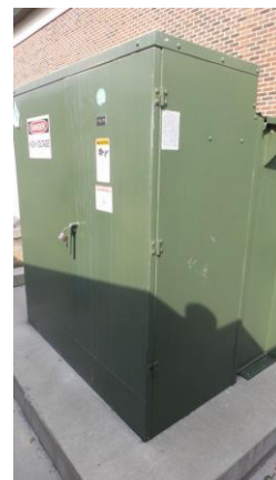
HSEL030e 4/21/2016 Transformer TX17 Ross Hall exterior
