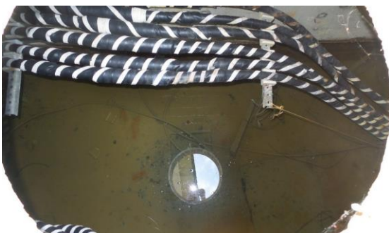
HSEL041e 4/21/2016 Standing water in manhole Between Brody and Life Sciences
