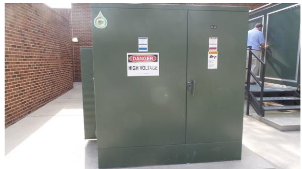
HSEL036e 4/21/2016 Oil-filled transformer TX-14 Family Medicine exterior
