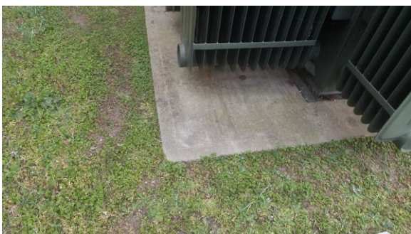
HSEL029e 4/21/2016 Transformer concrete slab settlement Allied Health exterior
