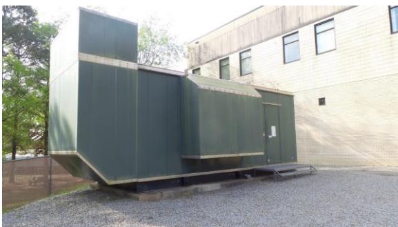
HSEL017e 4/21/2016 CUP emergency generator building Main substation
