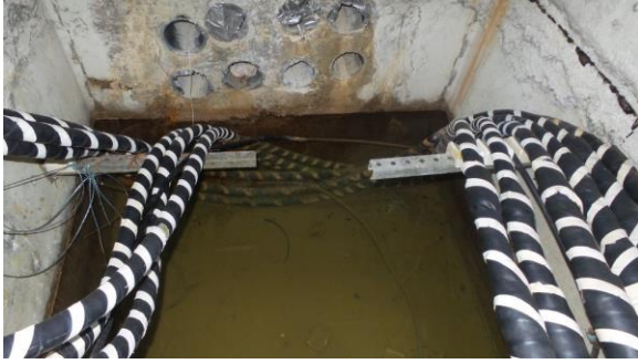
HSEL043e 4/21/2016 15 kV cable submerged in standing water Between Brody and Life Sciences
