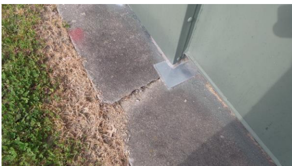
HSEL023e 4/21/2016 Damaged and repaired concrete slab Warren Life Sciences exterior
