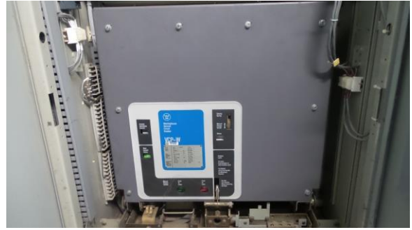
HSEL002e 4/21/2016 1,200 amp vacuum circuit breaker - SPARE GUC POD #2
