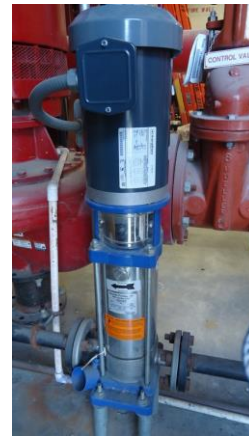
HSPWFP014e 3/8/2017 Inline centrifugal pump Central Plant
