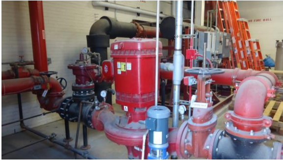
HSPWFP013e 3/8/2017 125 hp fire pump set-up Central Plant
