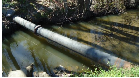
HSPWFP002e 3/8/2017 City-owned 15 inch ductile iron pipe crossing creek South side of West 5th Street
