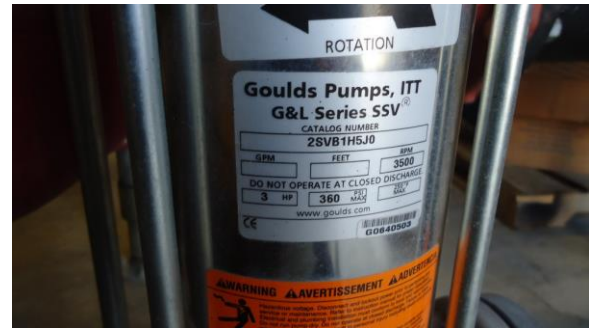
HSPWFP016e 3/8/2017 125 hp fire pump set-up Central Plant
