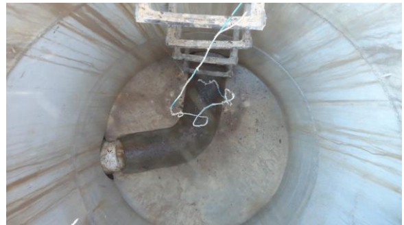
HSSANI010e 3/8/2017 Concrete manhole with minimal flow from one inlet Northwest corner of Family Medicine D4.1
