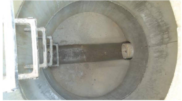
HSSANI008e 3/8/2017 Concrete manhole with minimal flow from one inlet North side of Family Medicine D4.1
