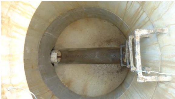
HSSANI009e 3/8/2017 Concrete manhole with minimal flow from one inlet North side of Family Medicine D4.1
