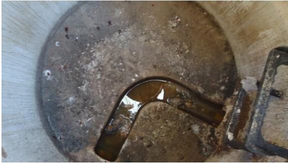
HSSANI007e 3/8/2017 Concrete manhole with low flow from one inlet Northeast corner of HSB C1.2
