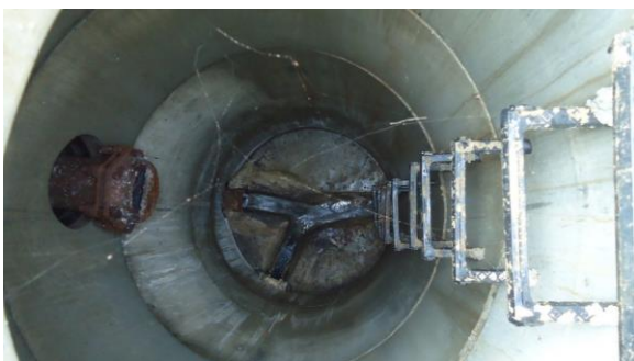
HSSANI011e 3/8/2017 Concrete manhole with moderate flow from two inlets Northwest side of Family Medicine D4.1
