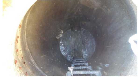
HSSANI002e 3/8/2017 Concrete manhole with significant flow from two inlets East side of Facilities Services C1.1
