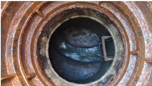
HSSANI003e 3/8/2017 Concrete manhole with metal rings and fast flow North side of Facilities Services C1.1
