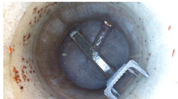
HSSANI006e 3/8/2017 Concrete manhole with moderate flow from two inlets East side of HSB in Health Sciences Drive C1.2
