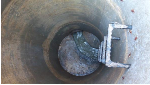
HSSANI001e 3/8/2017 Concrete manhole with significant flow from one inlet East side of Facilities Services C1.1
