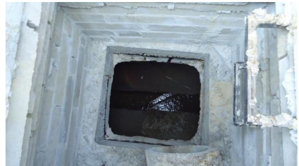
HSSANI004e 3/8/2017 Concrete manhole with flow from one inlet North Campus Drive by Biotechnology B1.2
