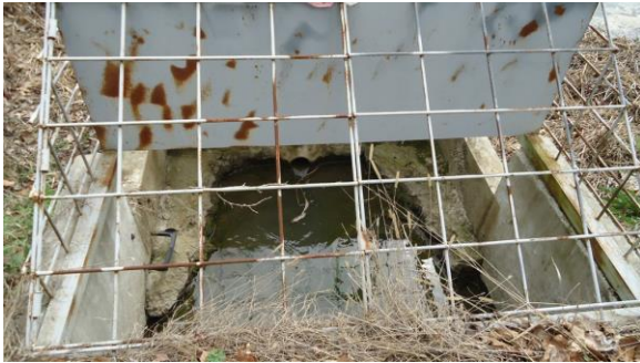
STRM027e 3/8/2017 Stormwater discharge structure Dental sch. stormwater management pond
