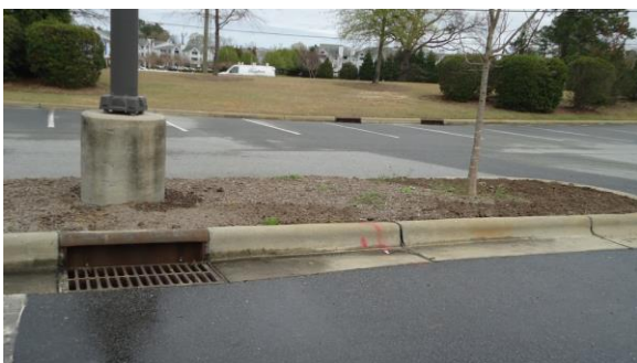
STRM017e 3/8/2017 Drainage inlet HSB northeast parking
