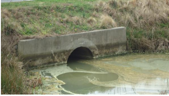
STRM025e 3/8/2017 Concrete headwall for 54 inch concrete pipe Dental sch. stormwater management pond
