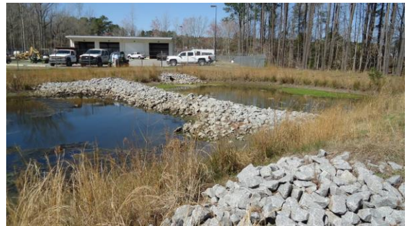
STRM052e 3/8/2017 Stormwater sediment control check dam Grounds stormwater management pond
