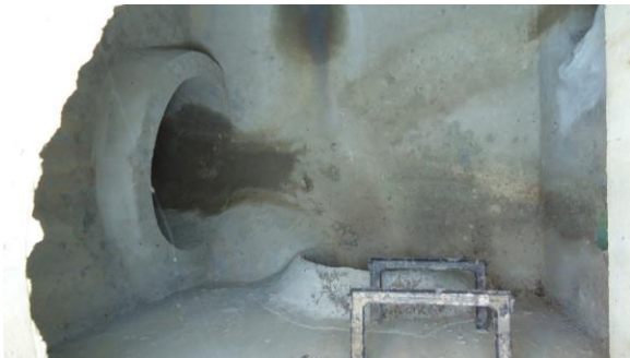
STRM063e 3/8/2017 Concrete stormwater manhole North of Family Medicine
