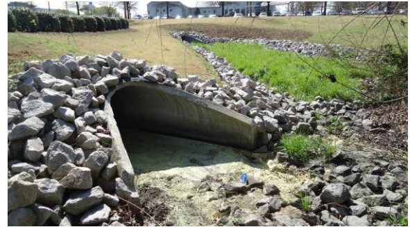
STRM046e 3/8/2017 Riprap-armored slope around 36 inch pipe outlet Southwest corner of Fam Med parking
