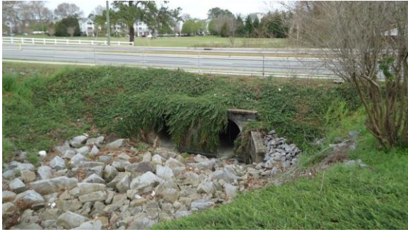
STRM013e 3/8/2017 Double 60 inch concrete pipe to carry lake flow north Under West 5th Street
