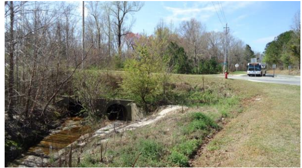
STRM040e 3/8/2017 Double 60 inch concrete pipe to carry lake flow northeast Under W Arlington to MacGregor Downs
