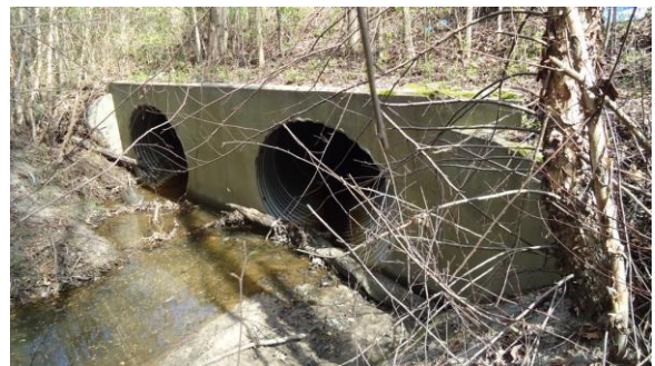
STRM042e 3/8/2017 Double 60 inch concrete pipe to carry lake flow northeast Under W Arlington to MacGregor Downs
