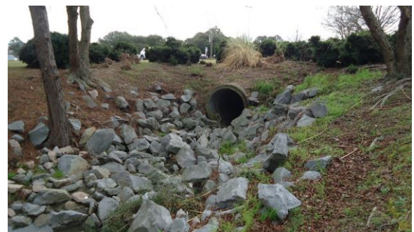
STRM006e 3/8/2017 Concrete headwall with 66 inch concrete pipe discharge South end of Lake Laupus by modular units
