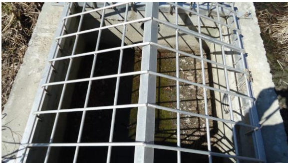
STRM051e 3/8/2017 Outlet structure Grounds stormwater management pond
