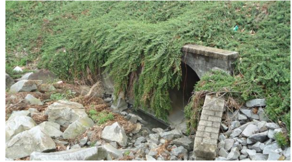
STRM014e 3/8/2017 Brick headwall and riprapped slope Under West 5th Street
