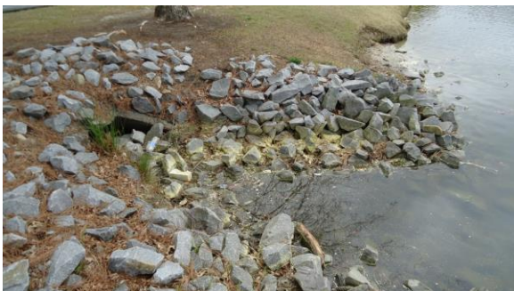
STRM011e 3/8/2017 Riprap-armored slope around pipe outlet with stone blocking outlet Lake Laupus northeast side
