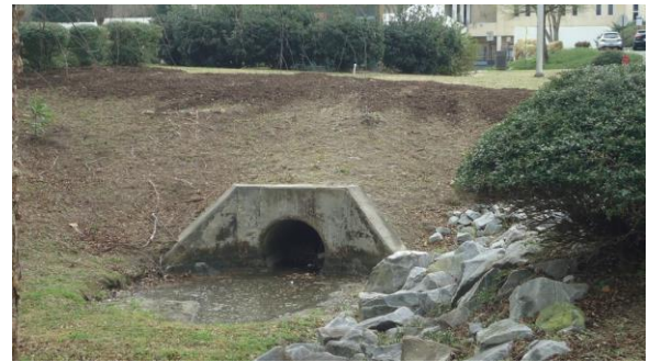
STRM004e 3/8/2017 Concrete headwall with 36 inch concrete pipe discharge South end of Lake Laupus
