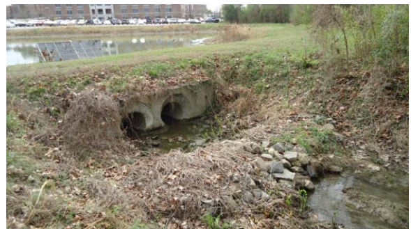
STRM030e 3/8/2017 Twin concrete discharge pipes Dental sch. stormwater management pond
