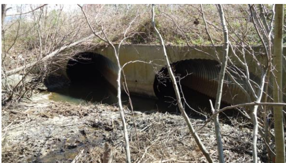
STRM053e 3/8/2017 Double 66 inch concrete pipes to carry flow northeast Under W Arlington to W 5th St
