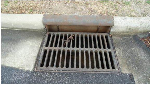
STRM019e 3/8/2017 Drainage inlet HSB north parking
