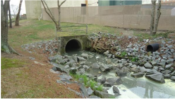
STRM001e 3/8/2017 Concrete headwall with 66 inch concrete pipe discharge South end of Lake Laupus by Facility Svcs
