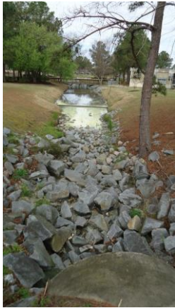
STRM007e 3/8/2017 Riprap-lined and filled drainage swale From pipe outlet toward Lake Laupus
