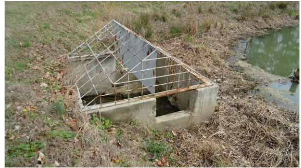
STRM028e 3/8/2017 Stormwater discharge structure Dental sch. stormwater management pond
