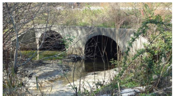
STRM054e 3/8/2017 Double 66 inch concrete pipes discharging flow northeast Under W Arlington to W 5th St
