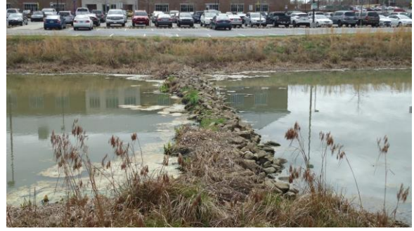
STRM026e 3/8/2017 Stormwater retention pond sediment control check dam Dental sch. stormwater management pond
