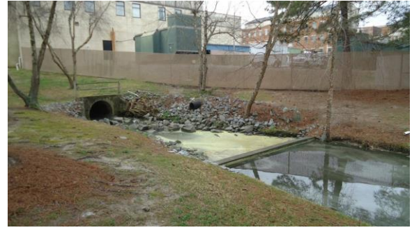
STRM002e 3/8/2017 Concrete headwall with 66 inch concrete pipe discharge South end of Lake Laupus by Facility Svcs
