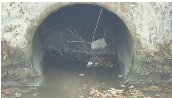
STRM005e 3/8/2017 36 inch pipe with outlet blockage South end of Lake Laupus
