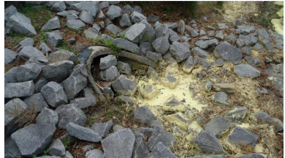
STRM010e 3/8/2017 Riprap-armored slope around pipe outlet with stone blocking outlet Lake Laupus northeast side
