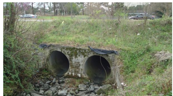
STRM018e 3/8/2017 Brick headwall for dual 66 inch pipe outfall from Lake Laupus Under West 5th Street
