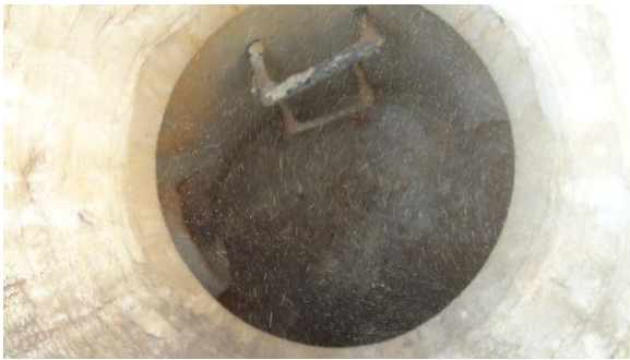
STRM069e 3/8/2017 Concrete stormwater manhole In parking just north of Dental
