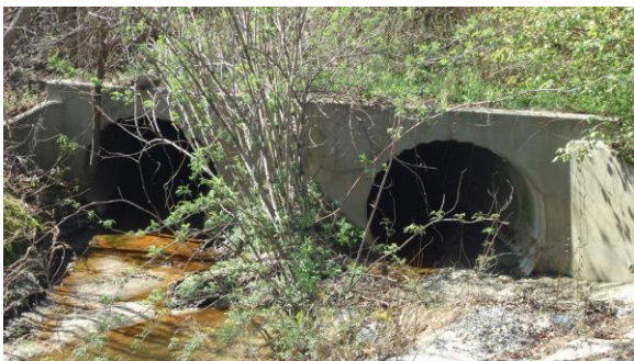
STRM041e 3/8/2017 Double 60 inch concrete pipe to carry lake flow northeast Under W Arlington to MacGregor Downs
