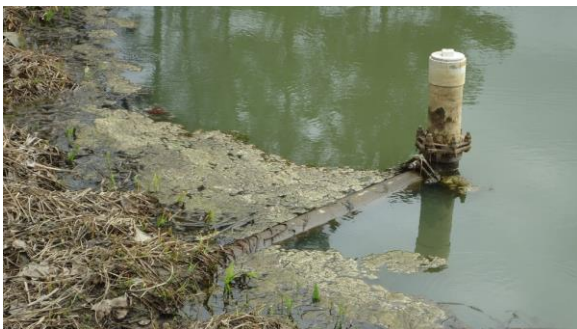
STRM029e 3/8/2017 Inlet control device Dental sch. stormwater management pond
