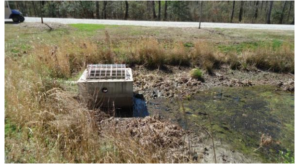
STRM050e 3/8/2017 Outlet structure Grounds stormwater management pond
