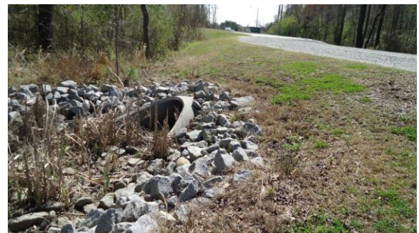
STRM048e 3/8/2017 Riprap-armored slope around 30 inch pipe outlet Under road leading to Grounds complex
