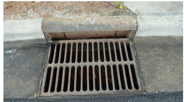
STRM016e 3/8/2017 Drainage inlet Health Sciences Drive
