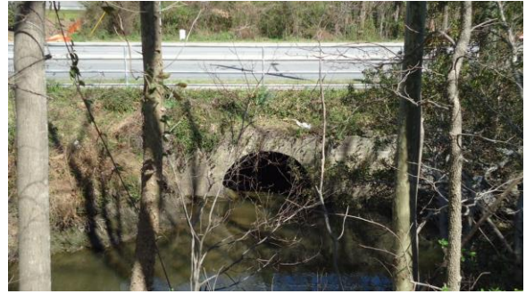
STRM056e 3/8/2017 Elliptical 4'x6' culvert to carry flow under road Under W 5th St to the north
