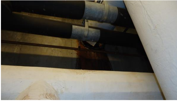
UTUN019e 4/21/2016 Evidence of past water infiltration around a pipe penetration through tunnel wall Interior of tunnel
