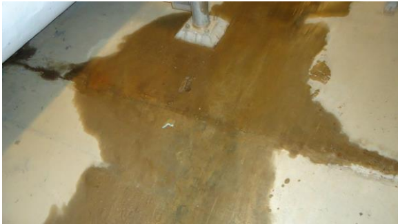
UTUN009e 4/21/2016 Moisture seeping up from floor joint Interior of tunnel
