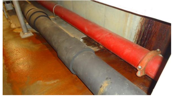
UTUN014e 4/21/2016 Evidence of past water infiltration around a pipe penetration through tunnel wall Interior of tunnel
