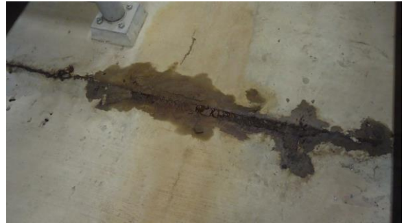
UTUN004e 4/21/2016 Moisture seeping up from floor joint Interior of tunnel
