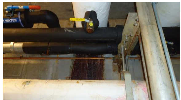
UTUN012e 4/21/2016 Evidence of past water infiltration around a pipe penetration through tunnel wall Interior of tunnel
