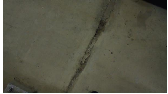
UTUN002e 4/21/2016 Previously repaired floor joint Interior of tunnel
