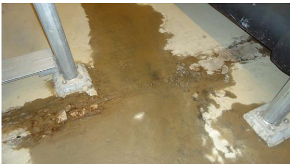
UTUN011e 4/21/2016 Previously repaired floor joint Interior of tunnel
