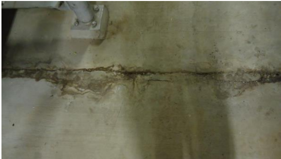
UTUN003e 4/21/2016 Previously repaired floor joint Interior of tunnel
