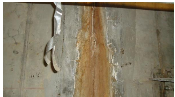
UTUN006e 4/21/2016 Evidence of past water infiltration through tunnel wall Interior of tunnel
