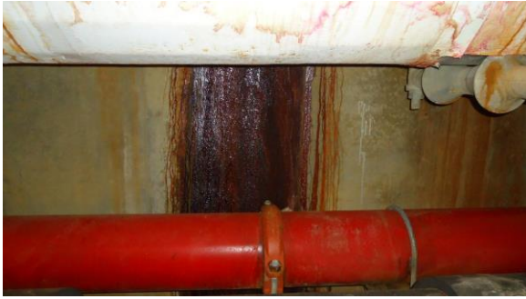
UTUN013e 4/21/2016 Evidence of past water infiltration around a pipe penetration through tunnel wall Interior of tunnel
