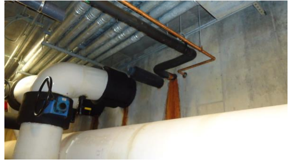
UTUN020e 4/21/2016 Evidence of past water infiltration around a pipe penetration through tunnel wall Interior of tunnel
