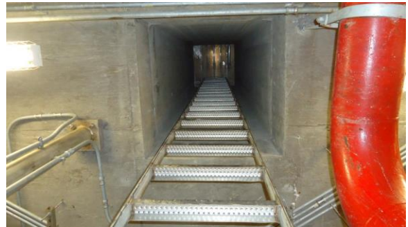
UTUN016e 4/21/2016 Emergency egress ladder and hatch Interior of tunnel
