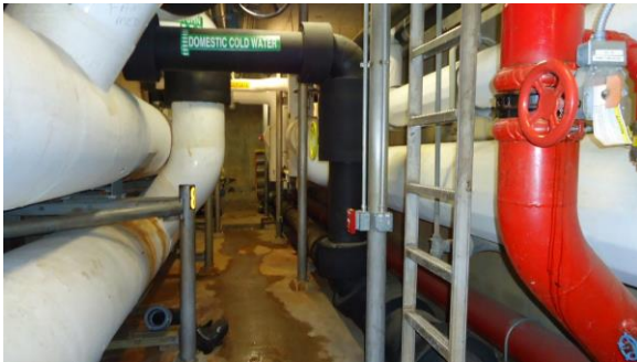
UTUN015e 4/21/2016 End of existing tunnel with emergency egress ladder Interior of tunnel
