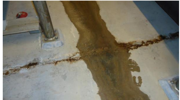
UTUN010e 4/21/2016 Moisture seeping up from floor joint Interior of tunnel
