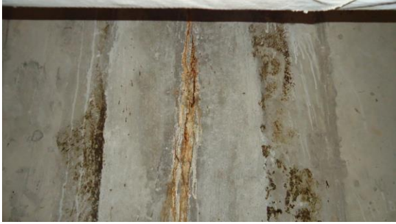
UTUN007e 4/21/2016 Evidence of past water infiltration through tunnel wall Interior of tunnel
