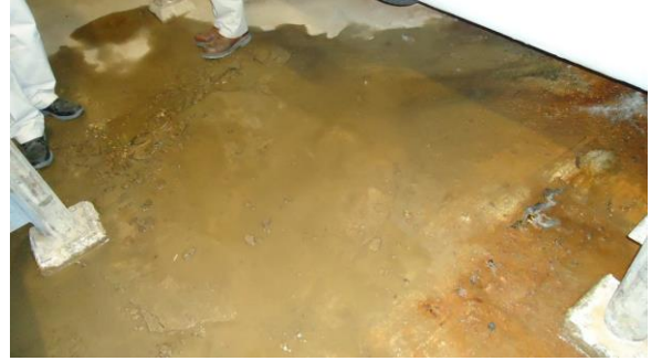
UTUN008e 4/21/2016 Accumulation of water on concrete floor of tunnel Interior of tunnel
