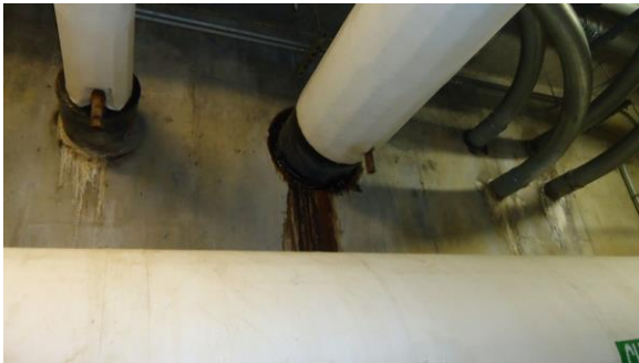
UTUN021e 4/21/2016 Evidence of past water infiltration around a pipe penetration through tunnel wall Interior of tunnel
