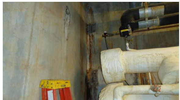
UTUN018e 4/21/2016 Stubbed out steam and chilled water lines for future expansion Interior of tunnel
