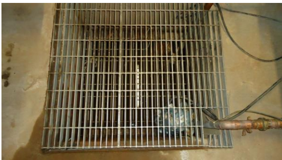
UTUN017e 4/21/2016 Metal grate over sump for collecting infiltration water and evacuating from tunnel Interior of tunnel
