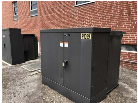
AUST041e 5/11/2021 Oil-filled transformer Site
