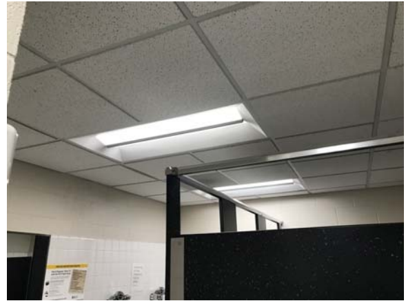
AUST004e 5/11/2021 Recessed LED lighting fixtures Third floor, restroom
