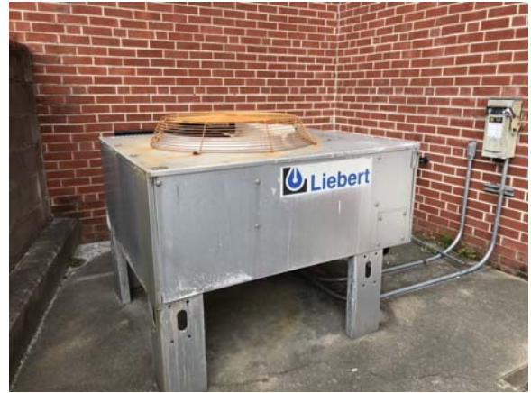
AUST022e 5/11/2021 Dry-cooler for computer AC unit Site
