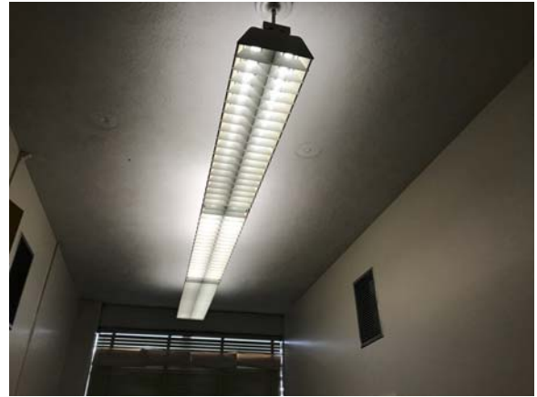
AUST007e 5/11/2021 Suspended T8 lighting fixtures Room 325B
