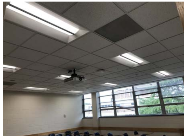
AUST003e 5/11/2021 Recessed LED lighting fixtures Room 321
