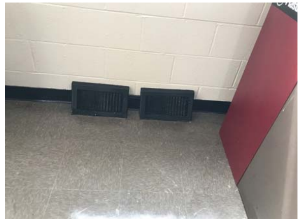
AUST006e 5/11/2021 HVAC diffusers Third floor corridor
