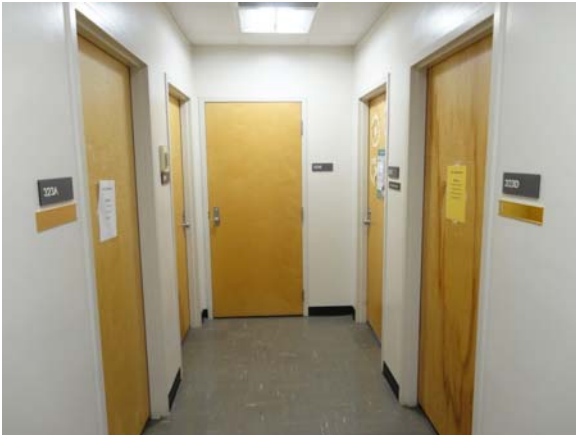
AUST017a 5/11/2021 Older doors with nonaccessible knob hardware Third floor, office suite
