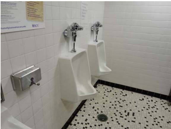
AUST009a 5/11/2021 Two wall-hung urinals Third floor, men's restroom
