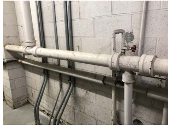
AUST019e 5/11/2021 Cast-iron piping with bell-and-spigot connections Room 144
