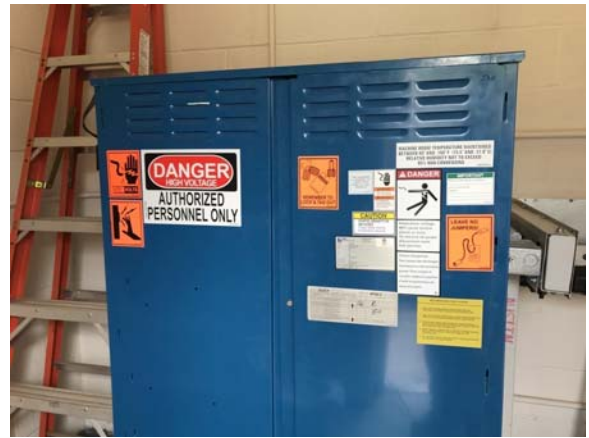
AUST043e 5/11/2021 Elevator controls Room 151
