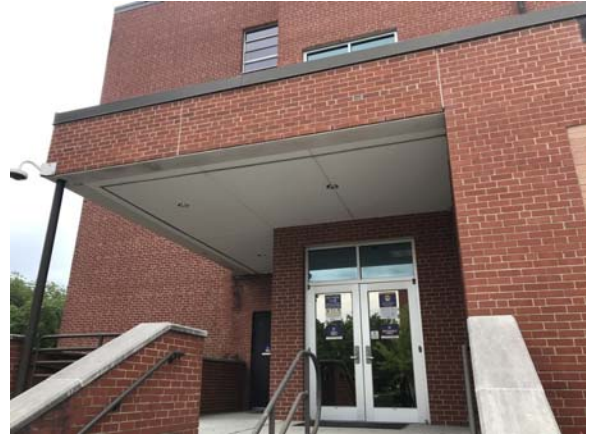
AUST044e 5/11/2021 Recessed can exterior lighting fixtures Soffit
