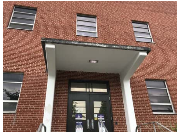
AUST020e 5/11/2021 Ceiling-mounted HID lighting fixture Entrance
