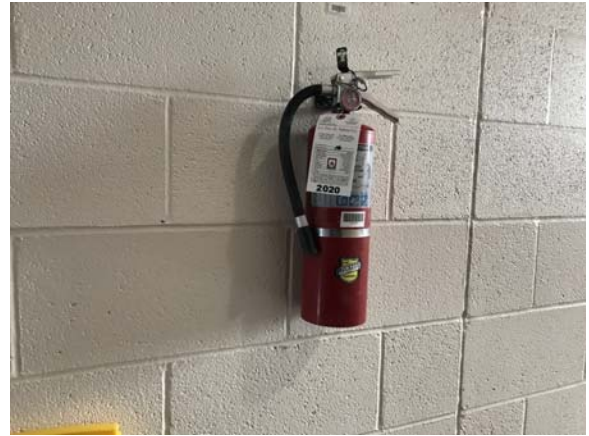
AUST008e 5/11/2021 Fire extinguisher Third floor corridor
