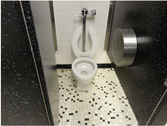
AUST010a 5/11/2021 Standard tankless water closet Third floor, men's restroom
