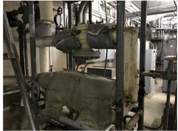
AUST037e 5/11/2021 Pressure reducing valves Room 149
