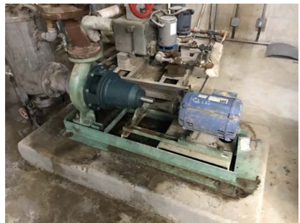
AUST030e 5/11/2021 Heating hot water pump Room 149
