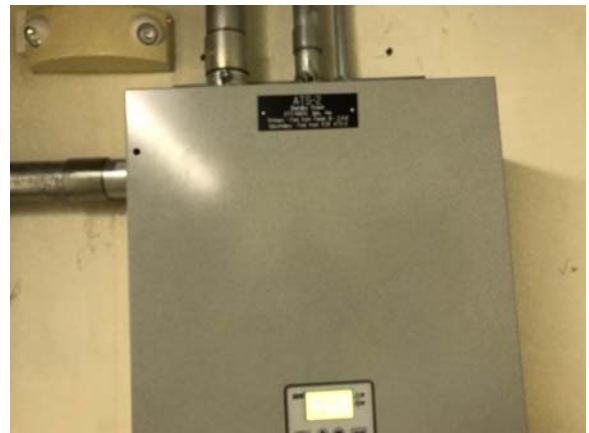
AUST039e 5/11/2021 Automatic transfer switch Room 149
