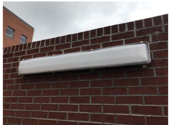
AUST024e 5/11/2021 Wall-mounted T8 lighting fixture Courtyard
