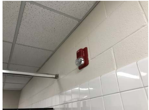
AUST005e 5/11/2021 Horn with strobe fire alarm device Third floor, restroom
