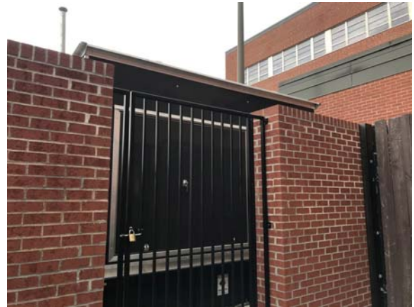
AUST023e 5/11/2021 Diesel-fired emergency generator Courtyard
