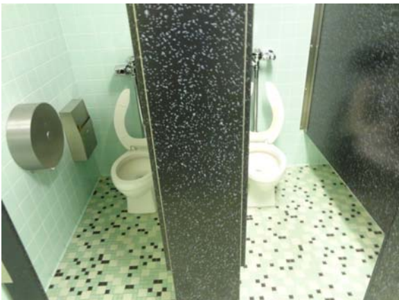
AUST015a 5/11/2021 Standard tankless water closet Third floor, women's restroom
