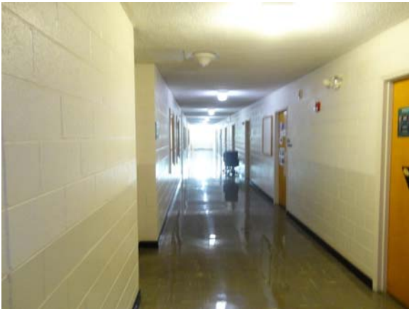
AUST029a 5/11/2021 Nine-inch vinyl floor tile, textured ceiling, and painted CMU walls Second floor corridor
