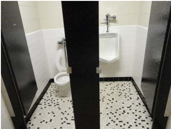
AUST020a 5/11/2021 Standard fixtures Third floor, men's restroom
