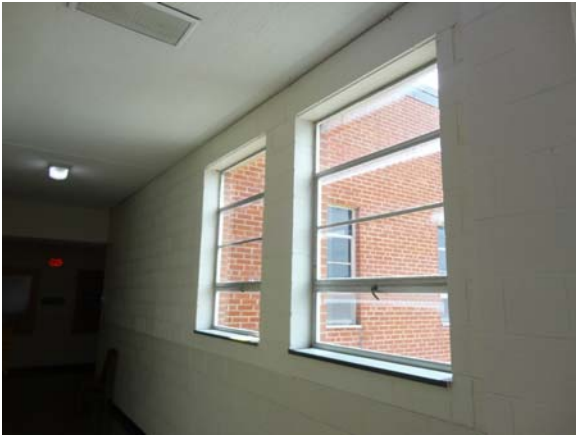
AUST013a 5/11/2021 Aging original single-pane, metal-framed windows Third floor corridor
