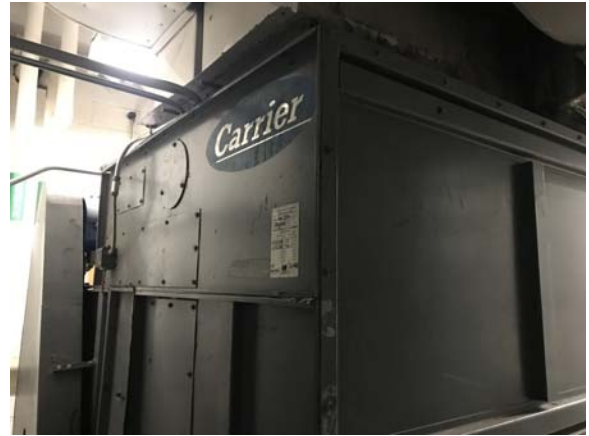
AUST013e 5/11/2021 Air handling unit AHU-003 Room 237
