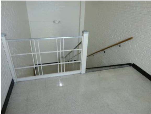
AUST004a 5/11/2021 Nonaccessible railing design Third floor, stair tower
