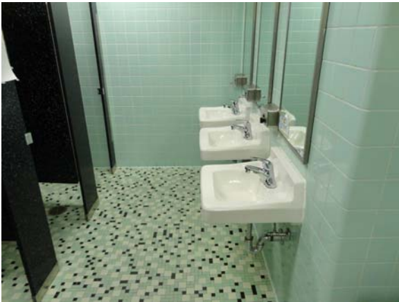
AUST014a 5/11/2021 Standard wall-hung lavatories Third floor, women's restroom
