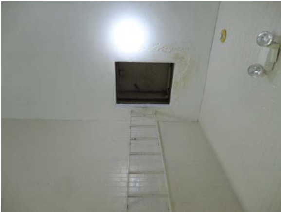
AUST002a 5/11/2021 Deteriorated roof access hatch and ladder Third floor, stair tower
