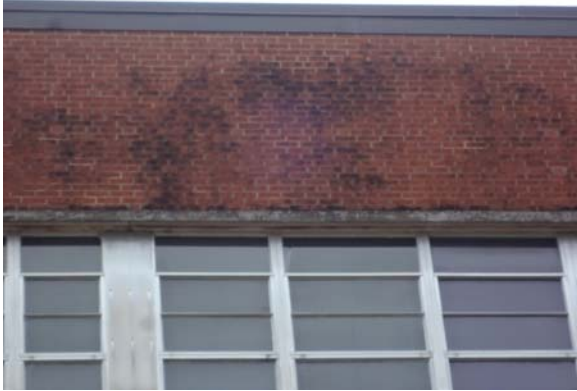
AUST047a 5/11/2021 Signs of upper masonry staining North elevation
