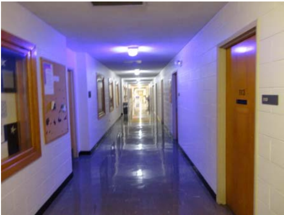
AUST032a 5/11/2021 Nine-inch vinyl floor tile, textured ceiling, and painted CMU walls First floor corridor
