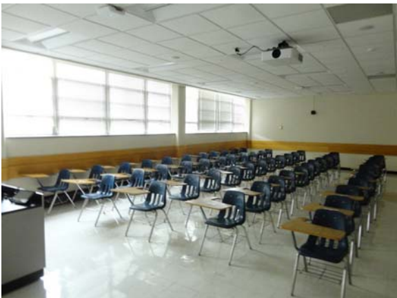
AUST039a 5/11/2021 Older vinyl composite floor tile and lay-in acoustical ceiling First floor, classroom
