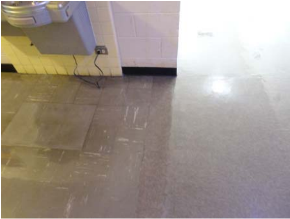
AUST028a 5/11/2021 Some dissimilar vinyl flooring repairs Second floor corridor
