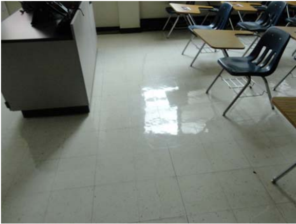
AUST040a 5/11/2021 Localized settlement crack in floor slab First floor, classroom
