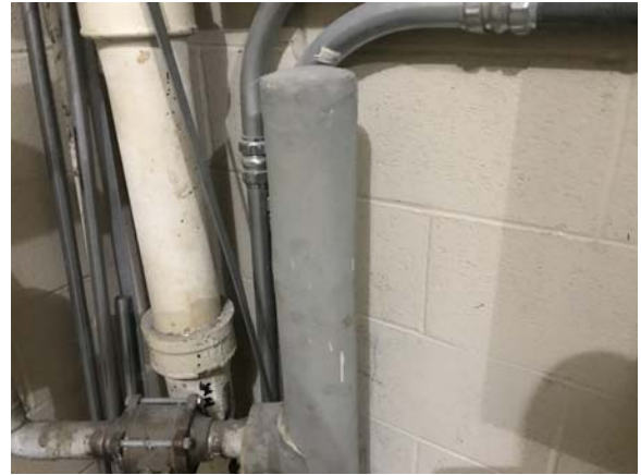
AUST010e 5/11/2021 Potential asbestos insulation on mechanical piping Room 336
