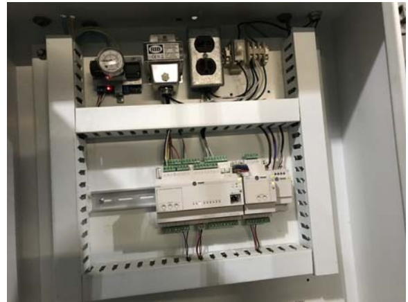
AUST032e 5/11/2021 HVAC field panel Room 149
