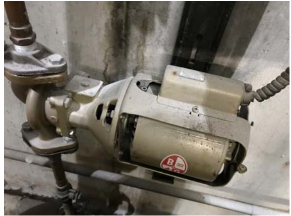
AUST034e 5/11/2021 Fractional horsepower domestic hot water pump Room 149
