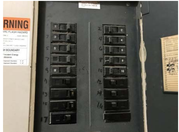
AUST002e 5/11/2021 Local panelboard Third floor corridor
