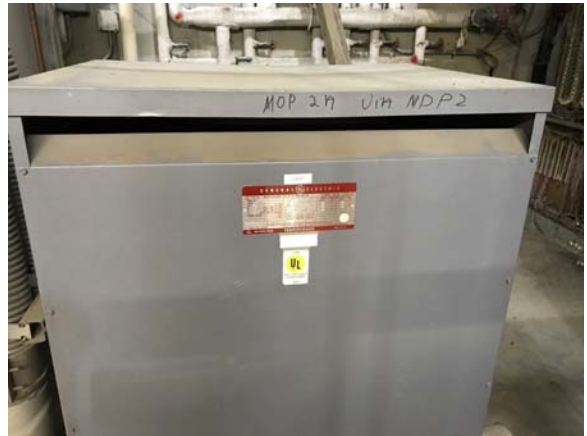
AUST035e 5/11/2021 Step-down transformer Room 149
