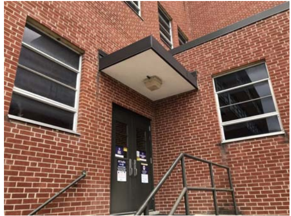
AUST040e 5/11/2021 Ceiling-mounted HID lighting fixture Entrance
