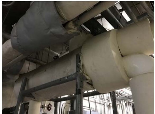
AUST036e 5/11/2021 Heating hot water shell-and-tube heat exchanger Room 149
