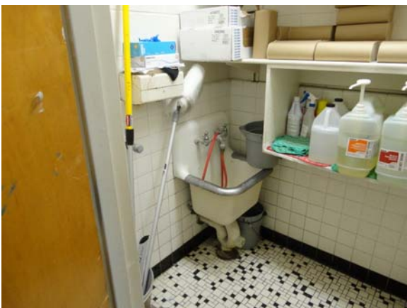
AUST030a 5/11/2021 Older wall-mounted service sink Second floor, janitor's closet
