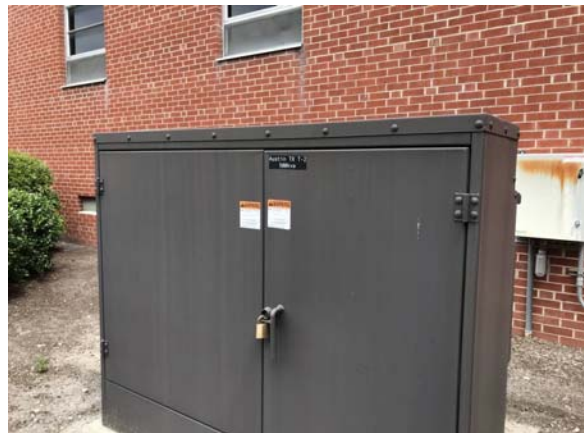
AUST042e 5/11/2021 Oil-filled transformer Site
