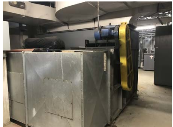
AUST027e 5/11/2021 Air handling unit AHU-001 Room 149
