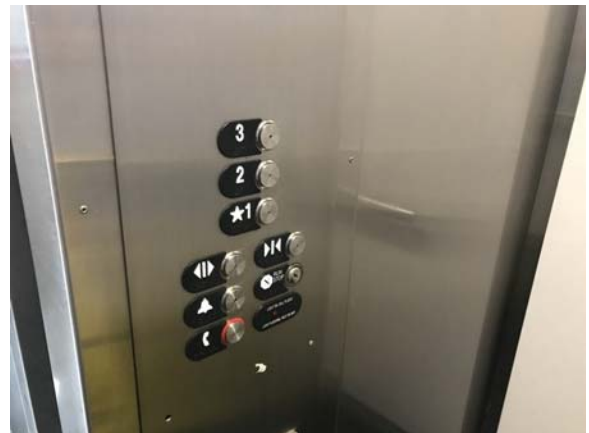
AUST012e 5/11/2021 Elevator control panel Elevator
