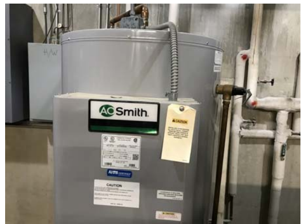
AUST033e 5/11/2021 Residential electric water heater Room 149
