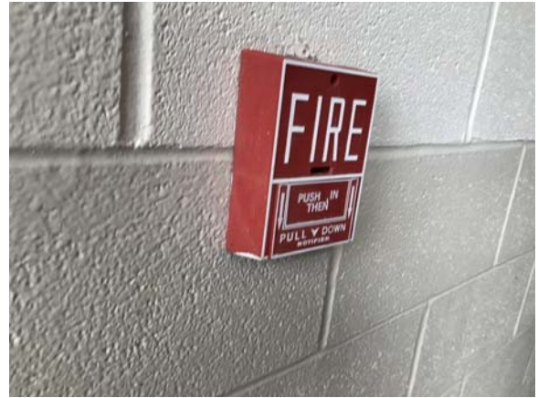
AUST001e 5/11/2021 Manual pull fire alarm device Third floor corridor
