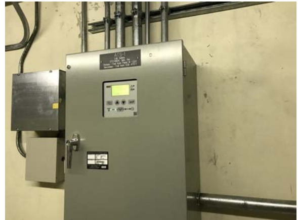
AUST038e 5/11/2021 Automatic transfer switch Room 149
