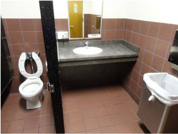
AUST037a 5/11/2021 Accessible counter sink First floor, women's restroom
