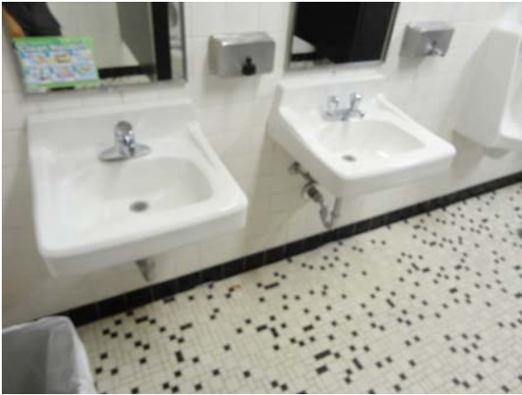
AUST008a 5/11/2021 Partially accessible wall-hung lavatories Third floor, men's restroom
