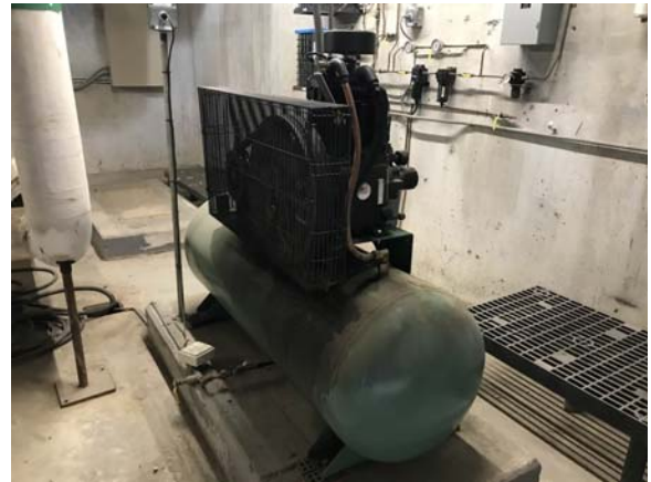
AUST026e 5/11/2021 Controls air compressor Room 149
