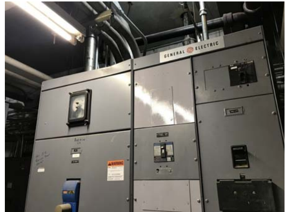
AUST029e 5/11/2021 Main switchboard Room 149
