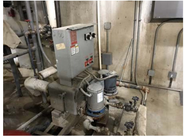
AUST031e 5/11/2021 Condensate receiver Room 149
