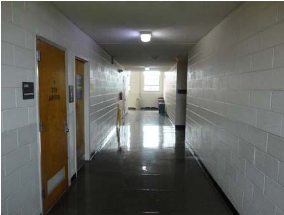
AUST007a 5/11/2021 Nine-inch vinyl floor tile, textured ceiling, and painted CMU walls Third floor corridor
