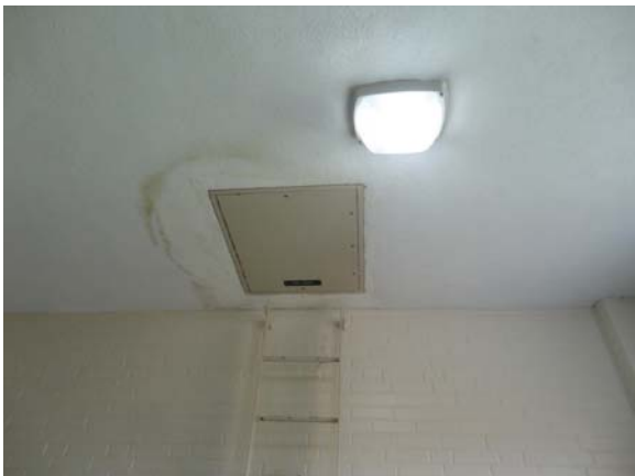
AUST003a 5/11/2021 A second deteriorated roof access hatch and ladder Third floor, stair tower
