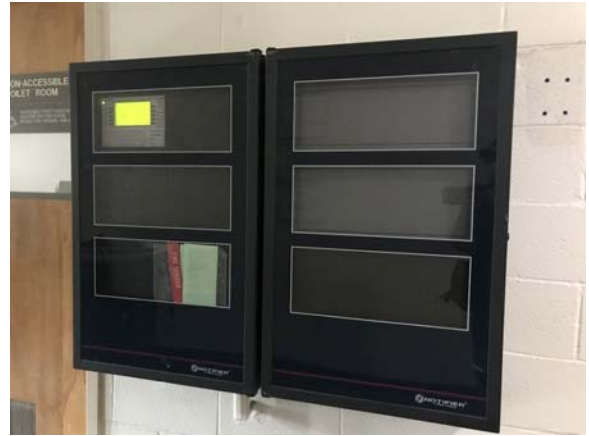
AUST016e 5/11/2021 Main fire alarm panel Room 144
