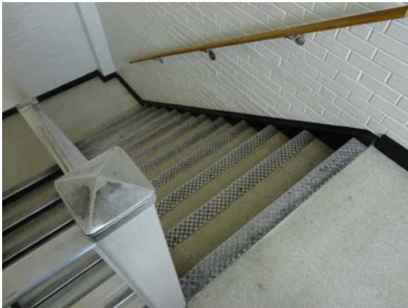
AUST005a 5/11/2021 Aging vinyl stair treads need upgrade Third floor, stair tower
