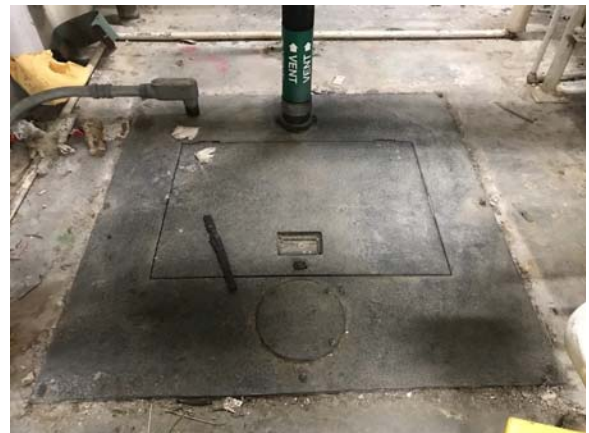
BATE024e 5/11/2021 Sump pump Room 1040A
