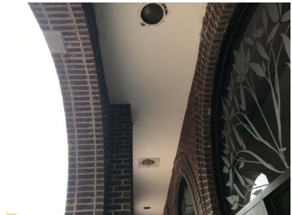
BATE039e 5/11/2021 Recessed can lighting fixtures Exterior
