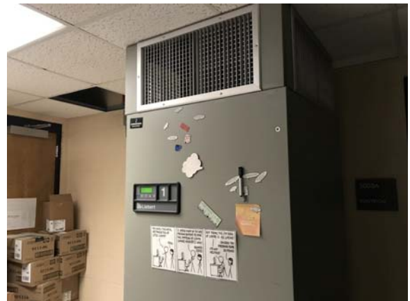
BATE018e 5/11/2021 Computer AC unit Room 3003
