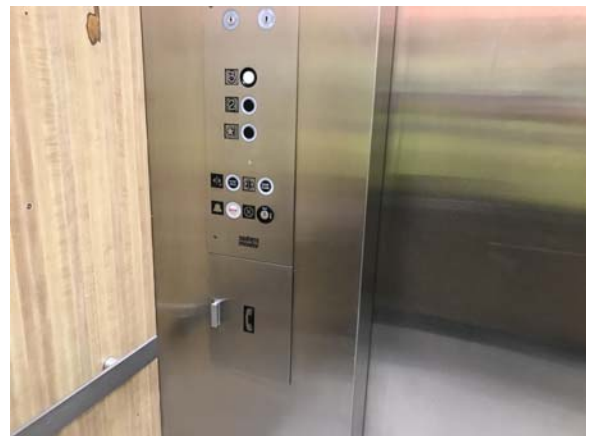
BATE012e 5/11/2021 Elevator interior Elevator 1
