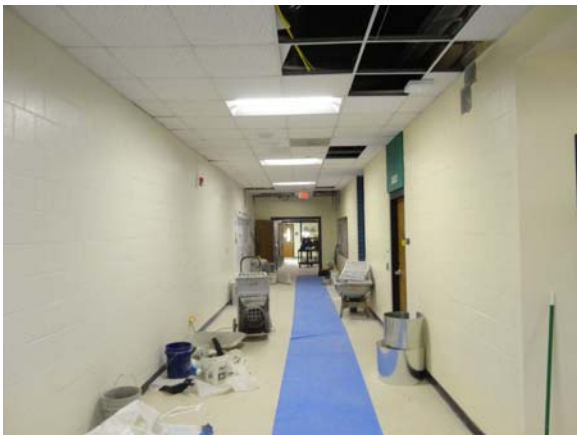
BATE006a 5/11/2021 Older VCT, acoustical ceiling, and painted block walls Third floor corridor
