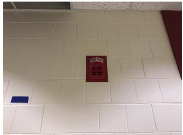
BATE015e 5/11/2021 Vintage horn with neon strobe fire alarm device Second floor corridor
