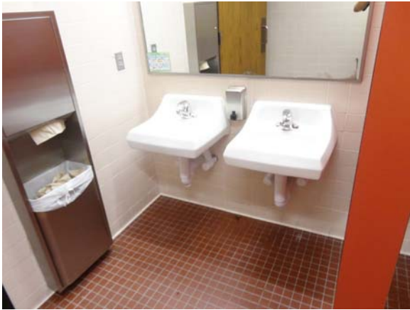
BATE019a 5/11/2021 Wall-hung lavatories Third floor, men's SE restroom
