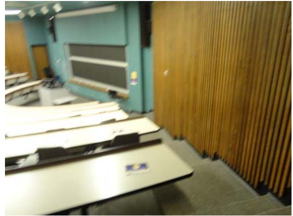
BATE050a 5/11/2021 No side aisle handrails First floor, larger tiered classroom
