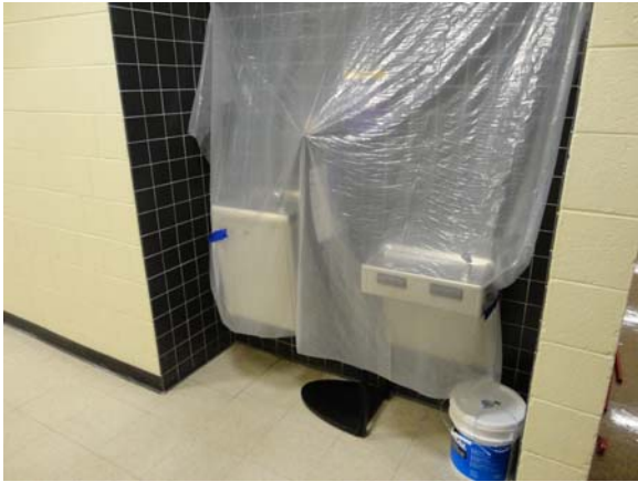
BATE010a 5/11/2021 Various ages of water fountains Third floor corridor
