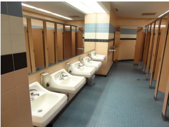
BATE030a 5/11/2021 Wall-hung lavatories Third floor, main women's restroom
