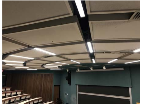
BATE016e 5/11/2021 LED lighting fixtures Room 1031
