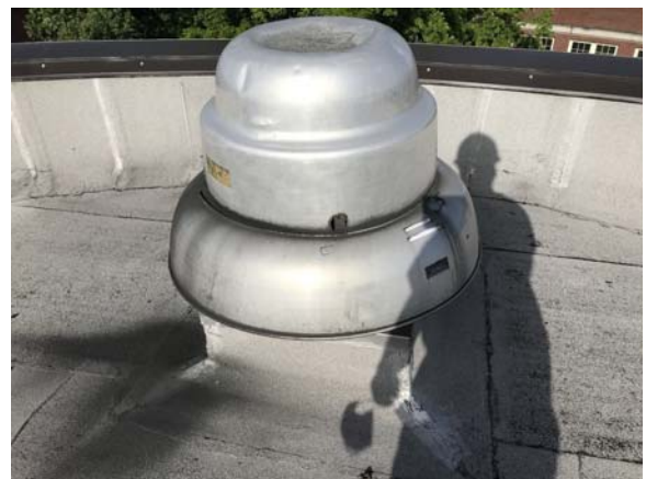
BATE003e 5/11/2021 Centrifugal rooftop exhaust fan Roof
