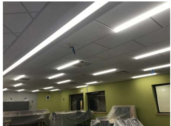
BATE006e 5/11/2021 LED lighting fixtures Room 3001
