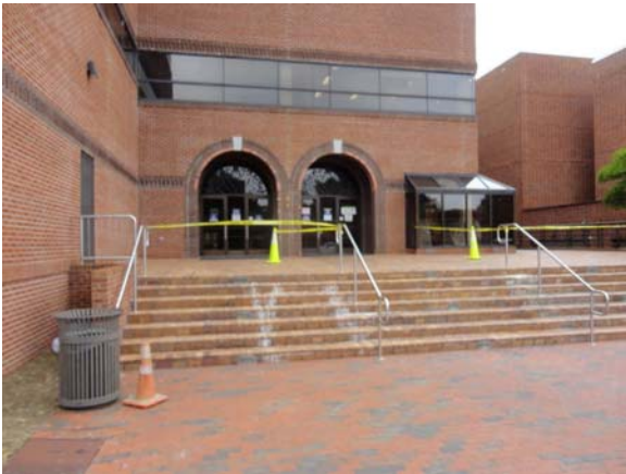
BATE069a 5/11/2021 Signs of efflorescence on plaza steps Southwest corner plaza
