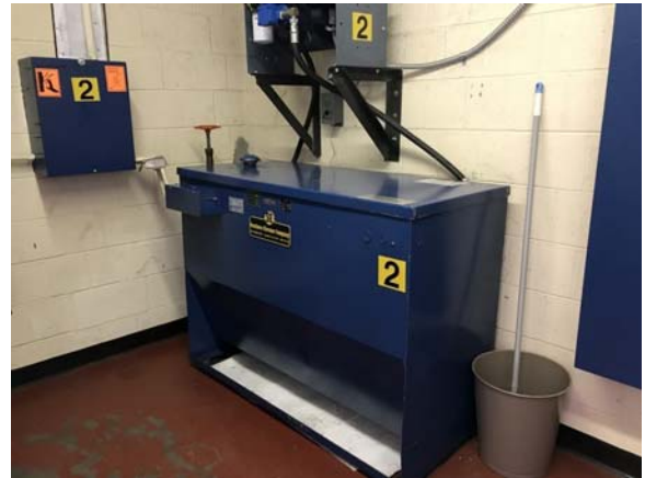
BATE041e 5/11/2021 Elevator 2 hydraulic controls Room 1036
