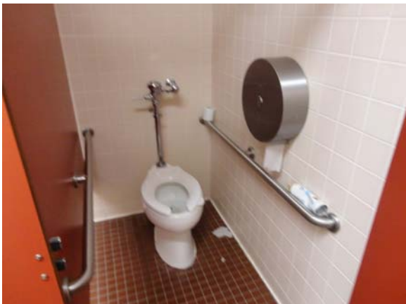
BATE021a 5/11/2021 Partially accessible toilet stall Third floor, men's SE restroom
