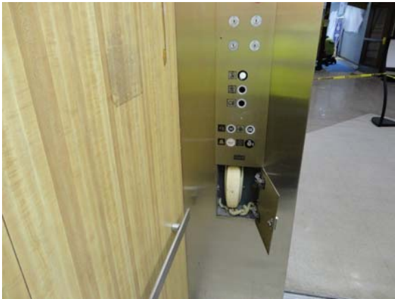
BATE038a 5/11/2021 Nonaccessible phone in elevator cab Passenger elevator cab
