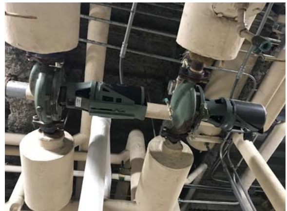
BATE021e 5/11/2021 Heating hot water pumps Room 1040A
