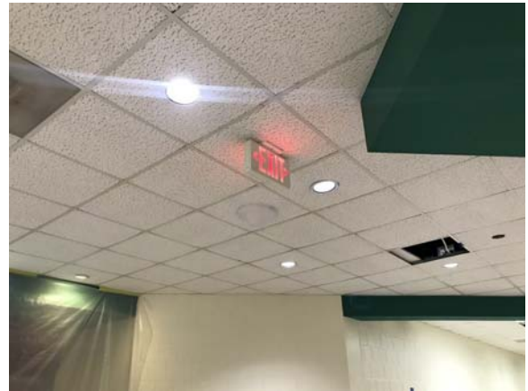
BATE014e 5/11/2021 Recessed can LED lighting fixtures Second floor, communal space
