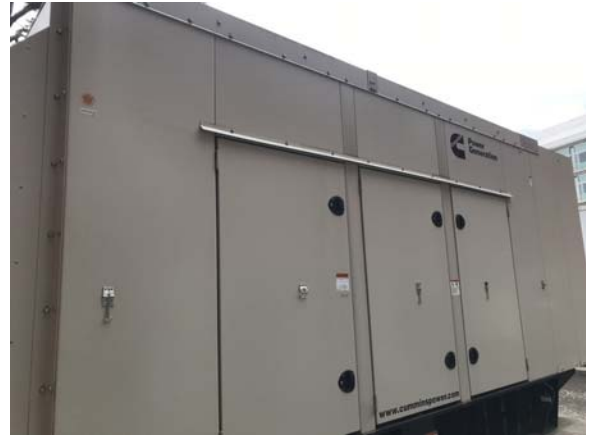
BATE034e 5/11/2021 Diesel-fired emergency generator Exterior
