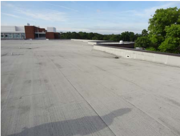
BATE002a 5/11/2021 Large, flat, built-up roof with low parapet wall and cap flashing Main roof
