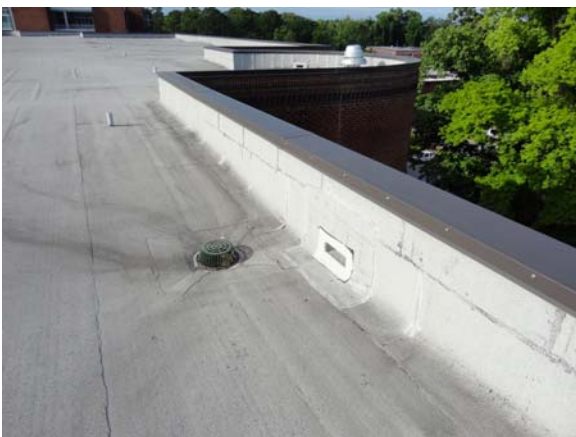
BATE003a 5/11/2021 Low perimeter parapet walls and metal cap flashing detail Main roof
