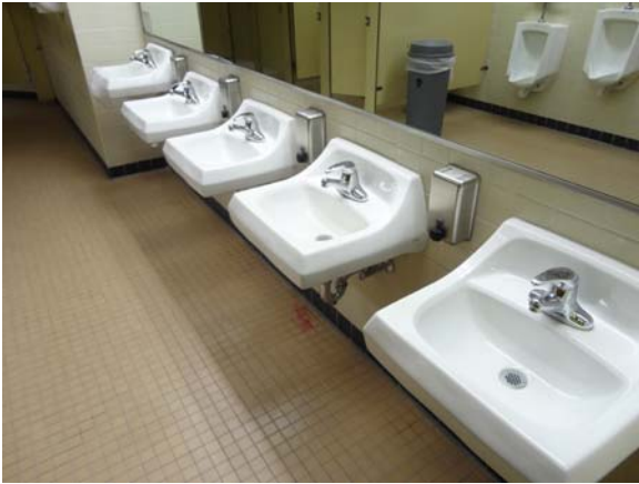
BATE034a 5/11/2021 Wall-hung lavatories Third floor, main men's restroom
