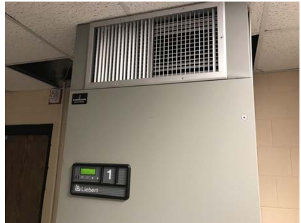
BATE017e 5/11/2021 Computer AC unit Room 3003
