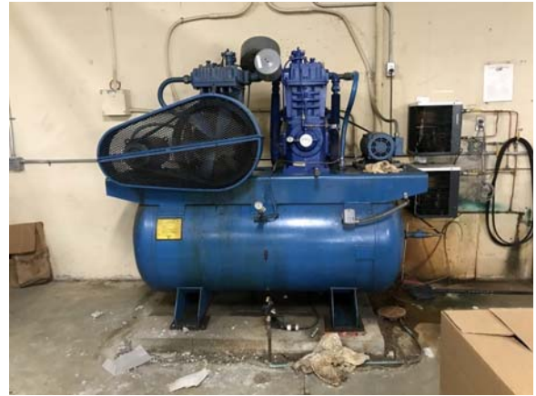
BATE031e 5/11/2021 Controls air compressor Room 1040A
