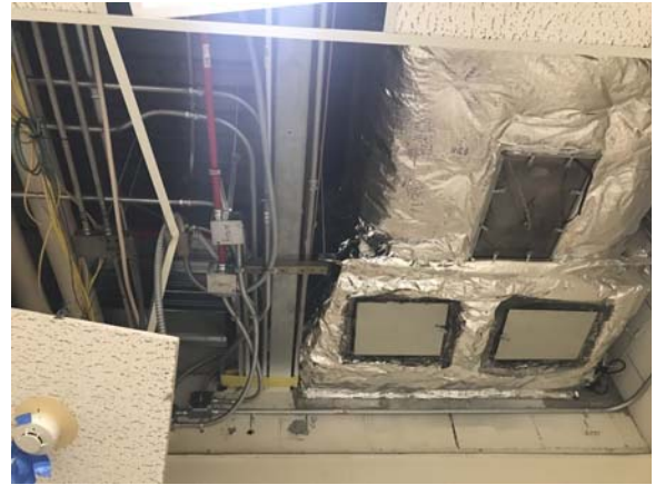
BATE010e 5/11/2021 Installation of new fire alarm and detection system and fire proofing Third floor corridor
