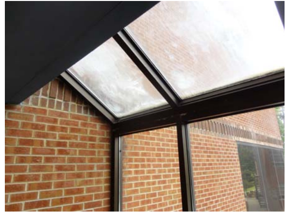
BATE056a 5/11/2021 Fogging on atrium glass First floor
