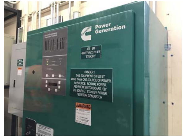
BATE037e 5/11/2021 Automatic transfer switch Room 1041
