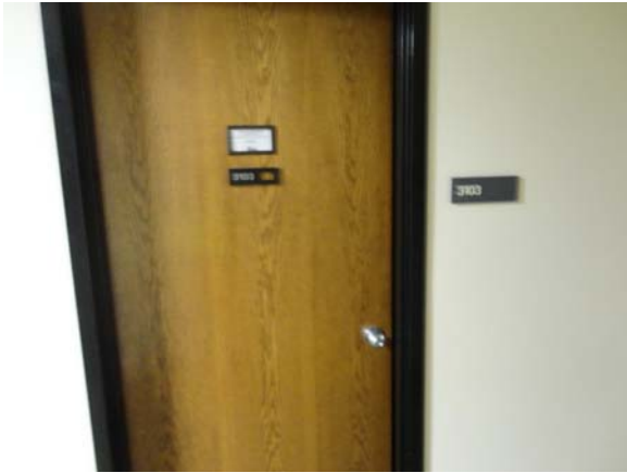
BATE016a 5/11/2021 Typical flush wood original door with knob hardware Third floor corridor
