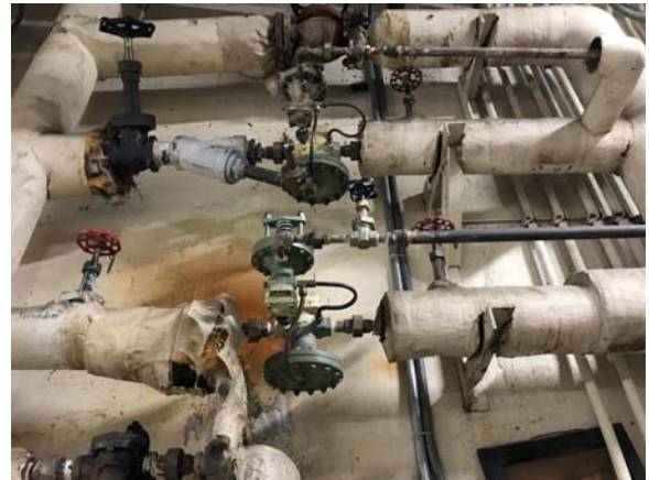
BATE023e 5/11/2021 Pressure reducing valves Room 1040A
