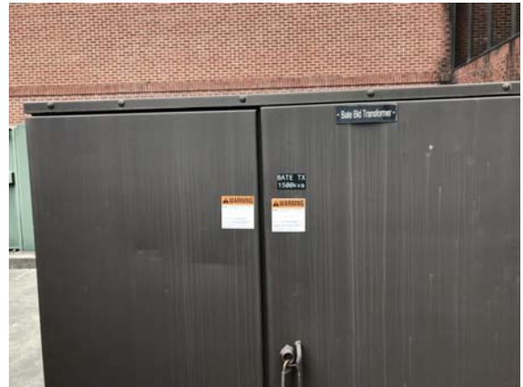
BATE032e 5/11/2021 Oil-filled transformer Site
