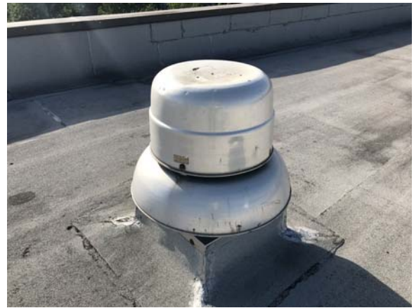
BATE004e 5/11/2021 Centrifugal rooftop exhaust fan Roof
