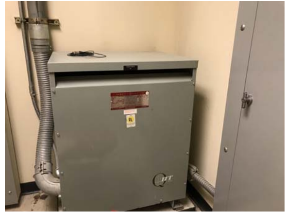
BATE007e 5/11/2021 Secondary step-down transformers Room 3103B
