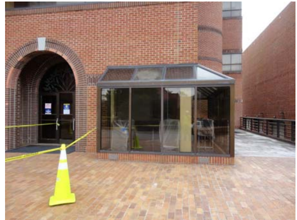
BATE070a 5/11/2021 Fogging on atrium glazing Southwest corner elevation
