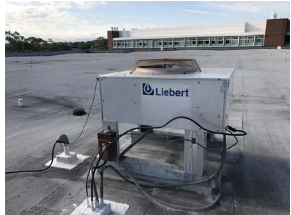
BATE002e 5/11/2021 Dry-cooler condensing unit for computer AC unit Roof
