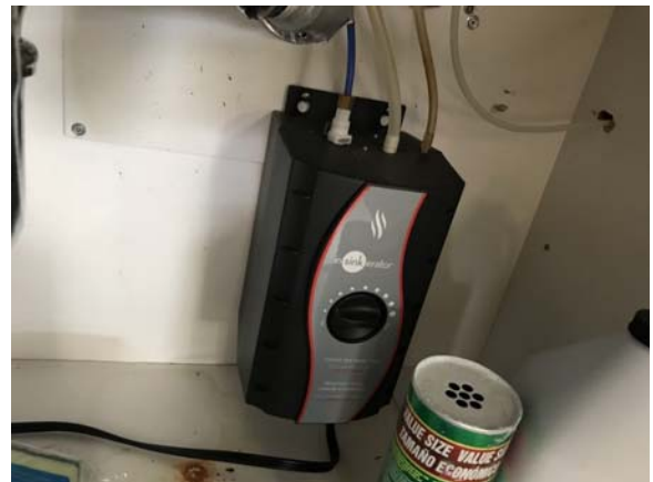
BATE009e 5/11/2021 Instantaneous electric water heater Room 3122
