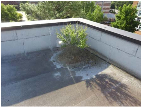
BATE005a 5/11/2021 Restricted roof drain Main roof
