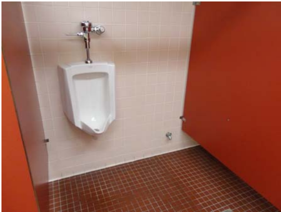
BATE020a 5/11/2021 Wall-hung urinal Third floor, men's SE restroom
