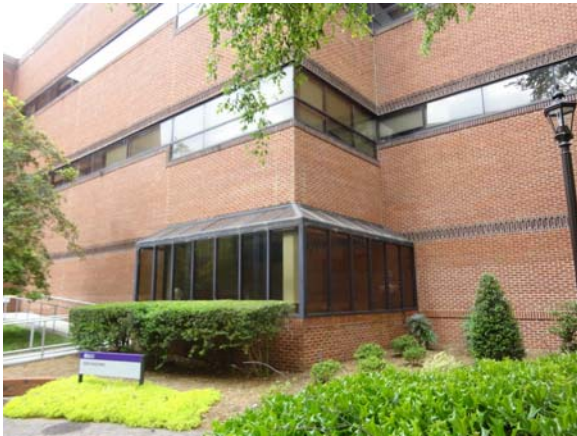
BATE063a 5/11/2021 Fogging atrium glazing Northeast elevation
