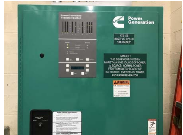
BATE038e 5/11/2021 Automatic transfer switch Room 1041
