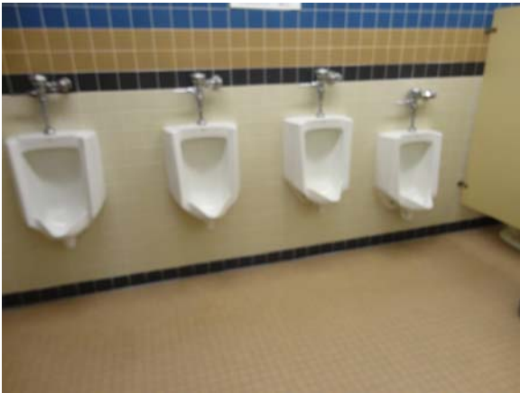
BATE035a 5/11/2021 Accessible wall-hung urinals Third floor, main men's restroom
