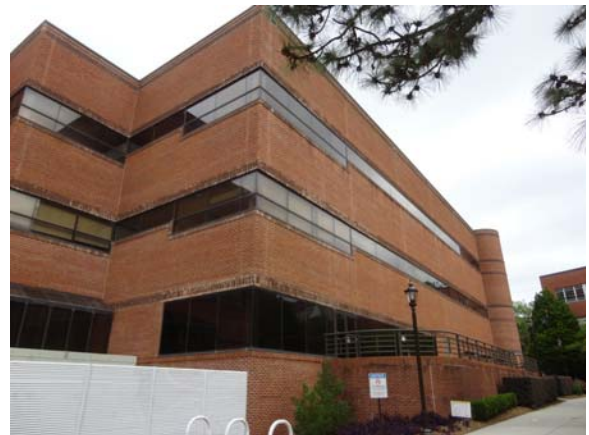
BATE060a 5/11/2021 Staining and streaking on exterior masonry South end of east elevation
