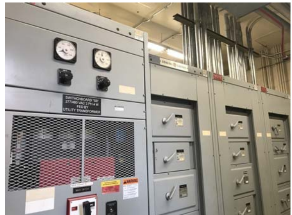
BATE036e 5/11/2021 Main switchboard Room 1041
