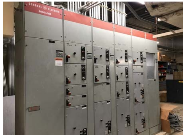
BATE030e 5/11/2021 Motor control center Room 1040A
