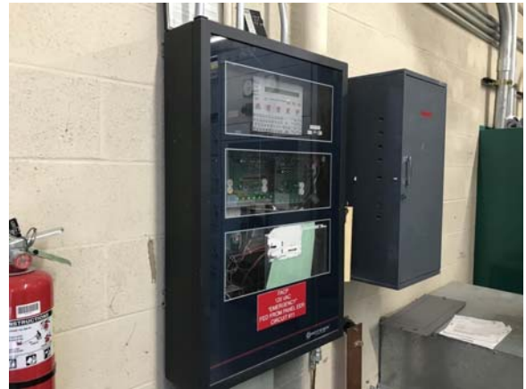
BATE035e 5/11/2021 Main fire alarm panel Room 1041
