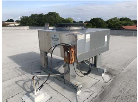
BATE001e 5/11/2021 Dry-cooler condensing unit for computer AC unit Roof
