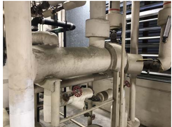
BATE020e 5/11/2021 Heating hot water shell-and-tube heat exchanger Room 1040A
