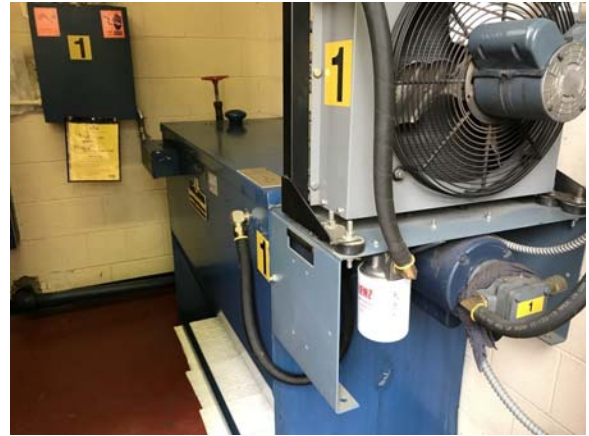
BATE040e 5/11/2021 Elevator 1 hydraulic controls Room 1036
