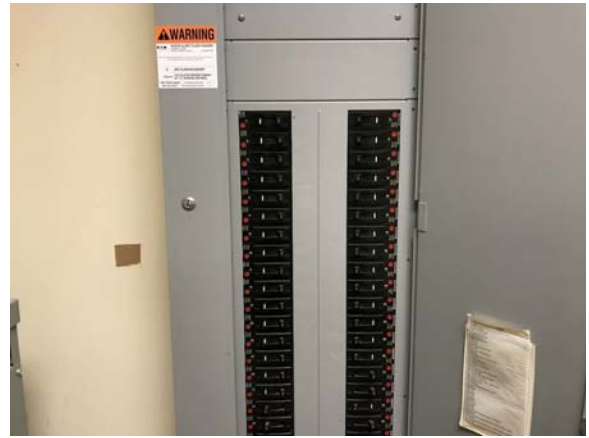
BATE008e 5/11/2021 Local panelboard Room 3103B
