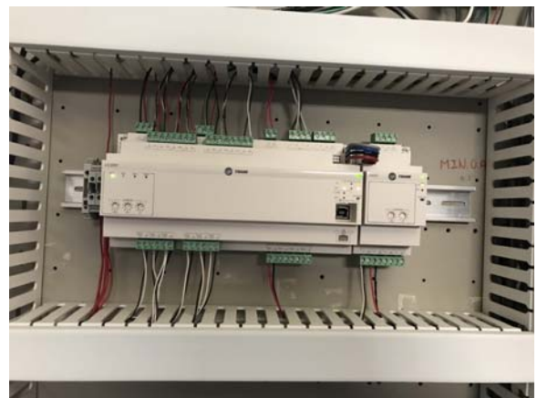
BREW018e 5/12/2021 HVAC field panel Room B209
