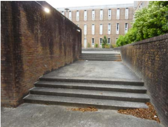
BREW081a 5/12/2021 No handrails on courtyard steps Central courtyard
