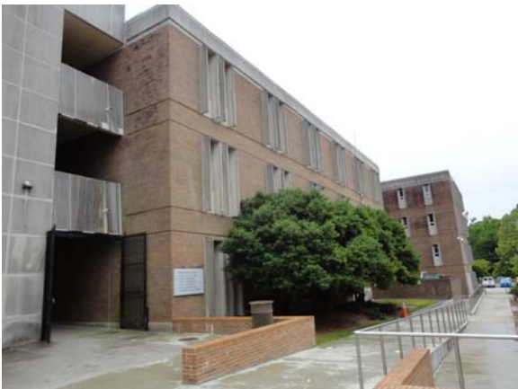
BREW083a 5/12/2021 Brick facade and stained cut stone facades East end of D Wing
