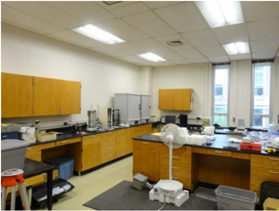
BREW061a 5/12/2021 Older VCT, older acoustical ceiling, and wood lab cabinet D Wing, second floor lab
