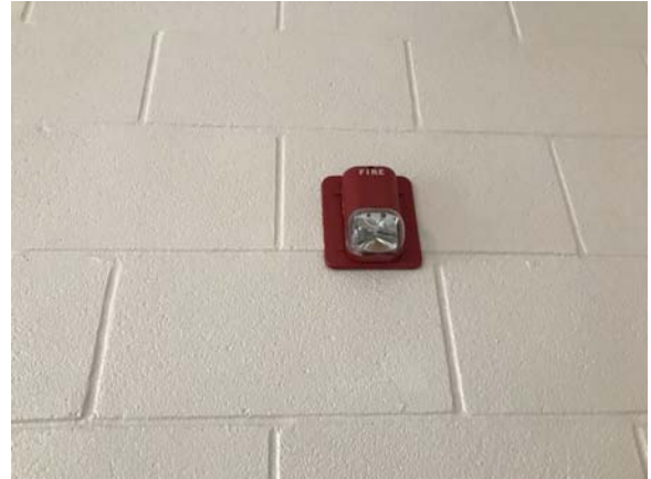
BREW011e 5/12/2021 Horn with strobe fire alarm device B Wing, third floor corridor
