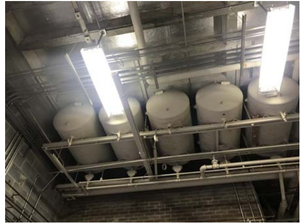
BREW034e 5/12/2021 Retrofitted LED lighting fixtures Room B109
