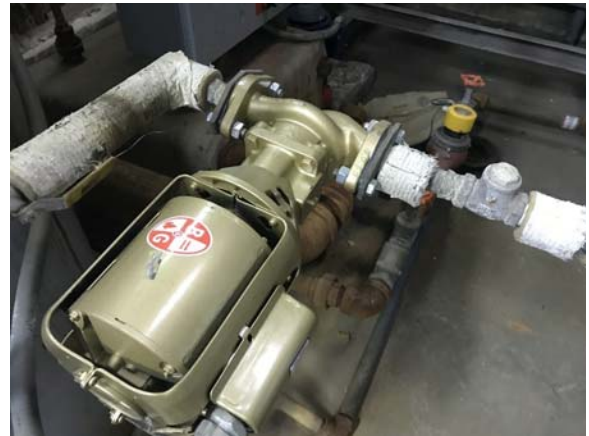
BREW029e 5/12/2021 Domestic hot water pump Room B109
