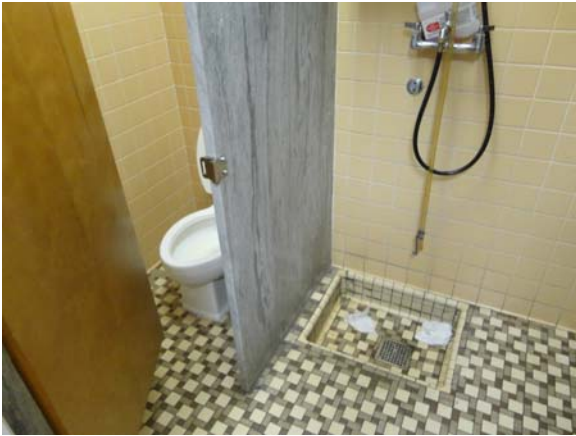
BREW028a 5/12/2021 Older standard water closet and floor mop sink B Wing, second floor janitor's closet
