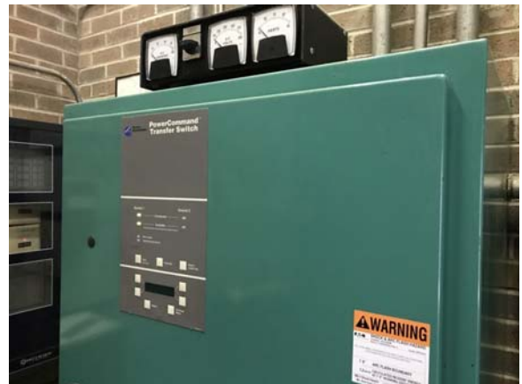
BREW036e 5/12/2021 Automatic transfer switch Room B109
