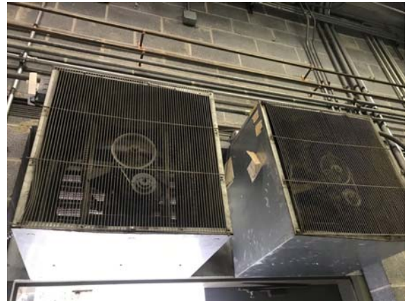
BREW023e 5/12/2021 Propeller exhaust fans Room B109
