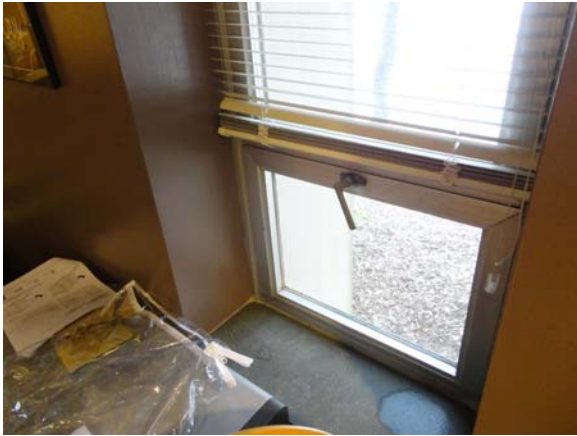
BREW043a 5/12/2021 Single-pane, original, metal-framed glazing D Wing
