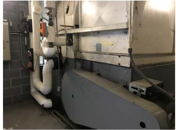
BREW019e 5/12/2021 Dual duct air handling unit Room B108
