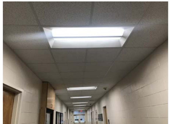
BREW015e 5/12/2021 Recessed LED lighting fixture B Wing, second floor corridor
