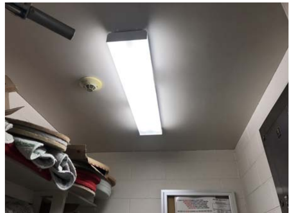
BREW042e 5/12/2021 Retrofitted LED lighting fixtures Room D110-3
