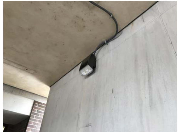
BREW014e 5/12/2021 LED scone lighting fixture Exterior stairwell
