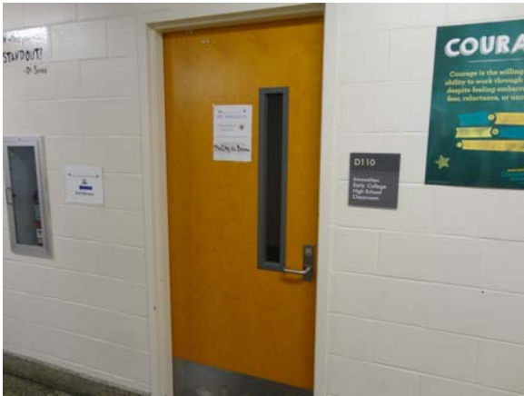
BREW041a 5/12/2021 Select newer corridor doors with lever hardware D Wing, first floor classroom
