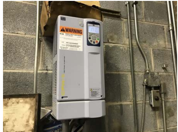
BREW038e 5/12/2021 VFD for heating hot water pump Room B109
