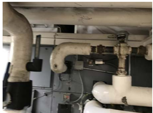
BREW063e 5/12/2021 Multizone air handling unit Room A445
