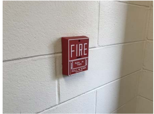
BREW013e 5/12/2021 Manual pull fire alarm device B Wing, third floor corridor
