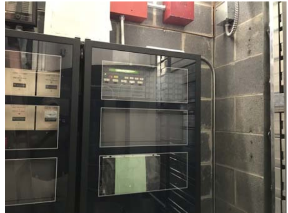
BREW062e 5/12/2021 Fire alarm extension panel Room C108
