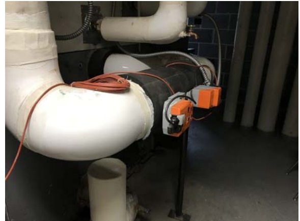
BREW055e 5/12/2021 DDC valve positioners Room C309
