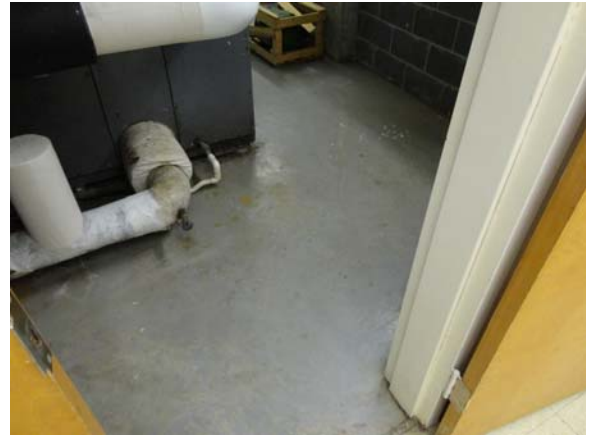
BREW074a 5/12/2021 Worn concrete sealer in typical mechanical room A Wing, third floor mechanical room
