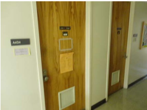
BREW072a 5/12/2021 Non-rated corridor doors with knob hardware A Wing, fourth floor corridor
