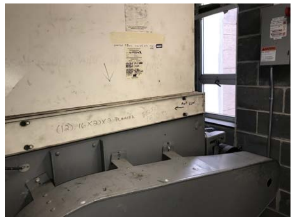
BREW057e 5/12/2021 Dual duct air handling unit Room C309
