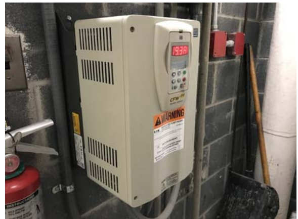
BREW048e 5/12/2021 VFD for air handling unit Room D219
