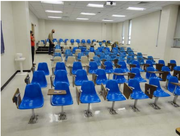
BREW065a 5/12/2021 Aging original fixed seating C Wing, first floor lecture room
