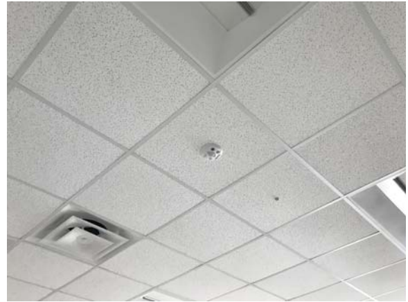
BREW010e 5/12/2021 Occupancy sensor and timing control Room B301
