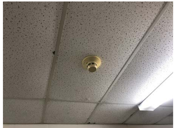
BREW012e 5/12/2021 Smoke detector and sagging ceiling tiles B Wing, third floor corridor
