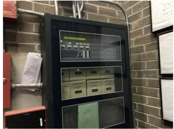
BREW037e 5/12/2021 Main fire alarm panel Room B109
