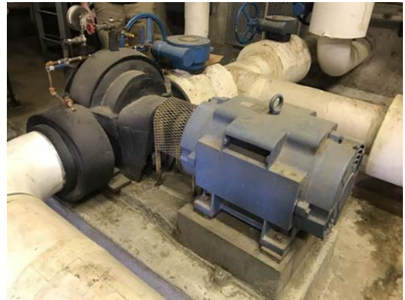
BREW026e 5/12/2021 Chilled water pump Room B109
