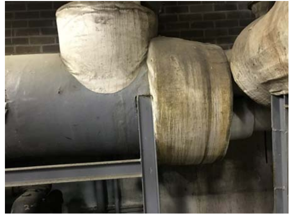
BREW031e 5/12/2021 Heating hot water shell-and-tube heat exchanger Room B109
