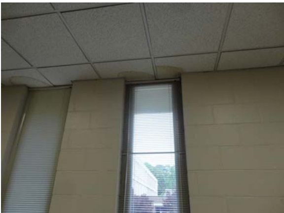
BREW066a 5/12/2021 Stained ceiling tile at window heads C Wing, first floor lecture room
