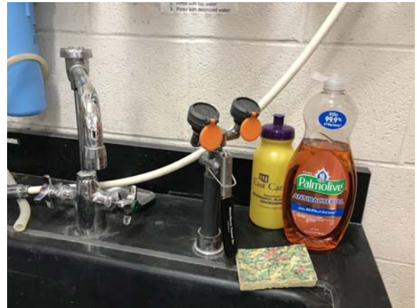
BREW053e 5/12/2021 Emergency eyewash Room D211
