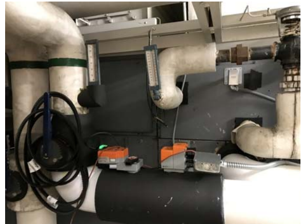
BREW065e 5/12/2021 Multizone air handling unit Room A345
