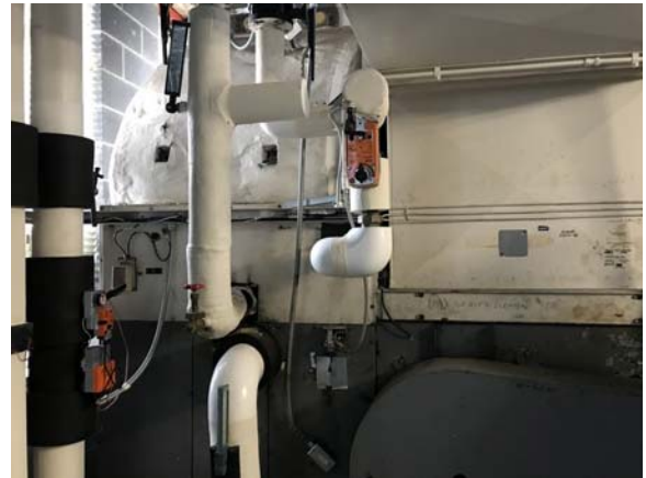
BREW008e 5/12/2021 Dual duct air handling unit Room B309
