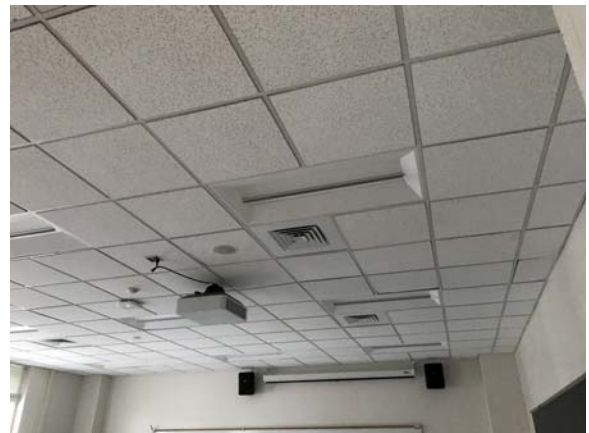
BREW054e 5/12/2021 Recessed LED lighting fixture Room C302
