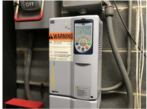
BREW070e 5/12/2021 VFD for air handling unit Room A139
