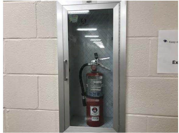
BREW043e 5/12/2021 Fire extinguisher D Wing, first floor corridor
