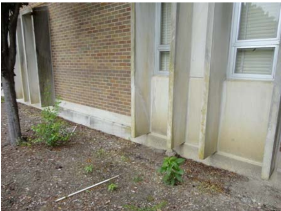
BREW089a 5/12/2021 Example of repaired stone solar fin South elevation of A Wing
