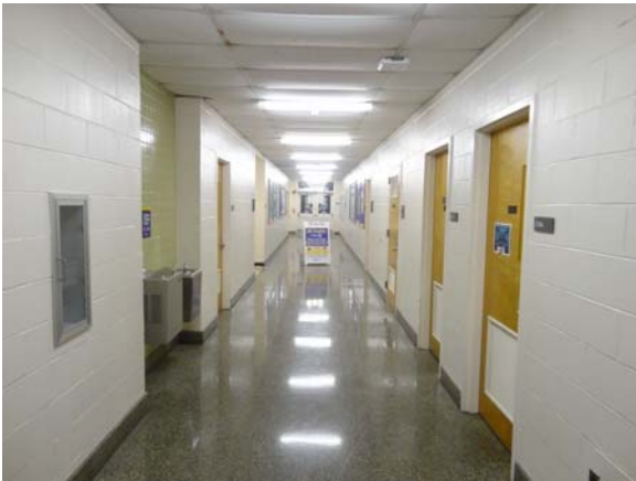
BREW062a 5/12/2021 Worn terrazzo, sagging acoustical ceiling, and painted CMU C Wing, second floor corridor
