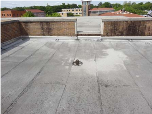
BREW007a 5/12/2021 Weathered built-up roof with cap sheet Brezeway roof
