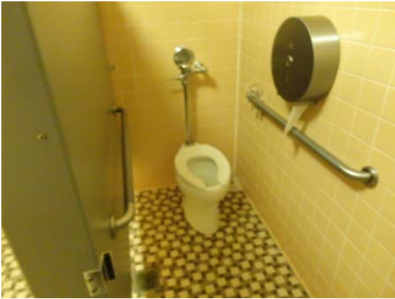
BREW031a 5/12/2021 Partially accessible toilet stall B Wing, first floor men's restroom
