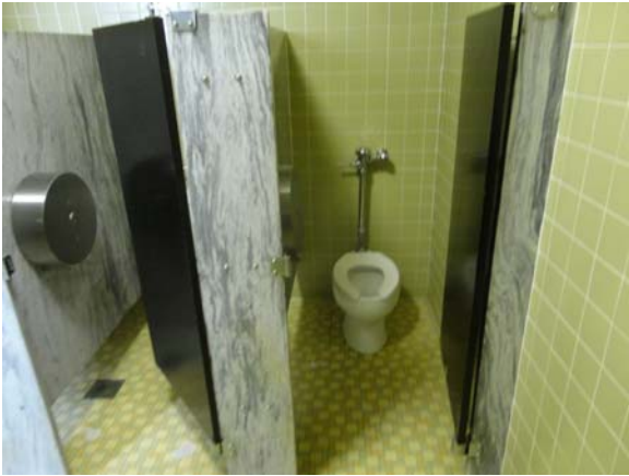
BREW022a 5/12/2021 Standard tankless water closet B Wing, third floor women's restroom
