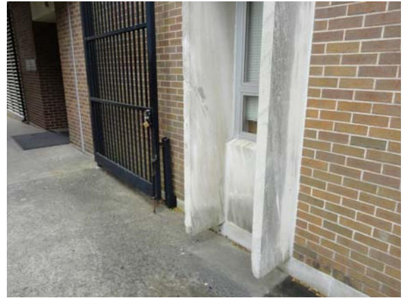
BREW092a 5/12/2021 Courtyard gates have padlocks without emergency egress Typical courtyard gate
