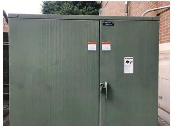
BREW020e 5/12/2021 Oil-filled transformer B Wing site
