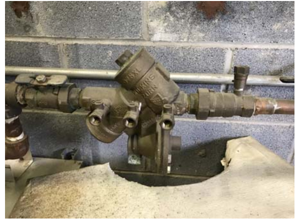
BREW022e 5/12/2021 Backflow preventer Room B109
