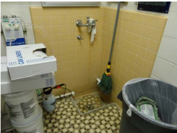
BREW039a 5/12/2021 Aging, original janitor's sink D Wing, first floor janitor's closet
