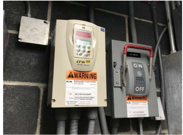
BREW061e 5/12/2021 VFD for air handling unit Room C208
