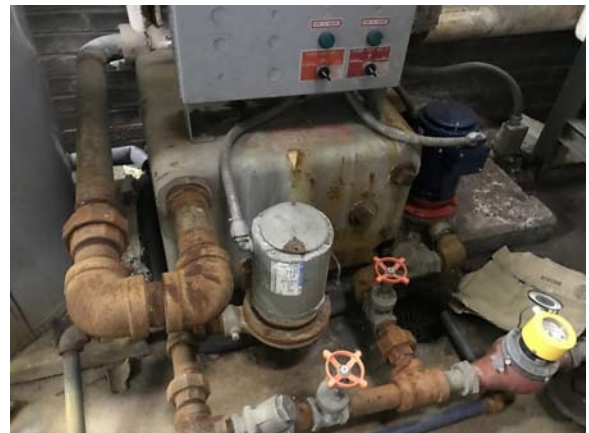
BREW030e 5/12/2021 Condensate receiver Room B109
