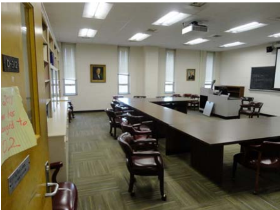
BREW054a 5/12/2021 Newer carpet tile and acoustical ceiling D Wing, third floor conference room
