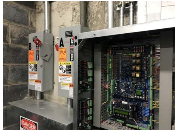
BREW041e 5/12/2021 Elevator controls Room B117
