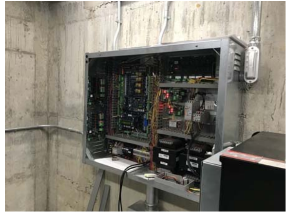
BREW040e 5/12/2021 Elevator controls Room B117
