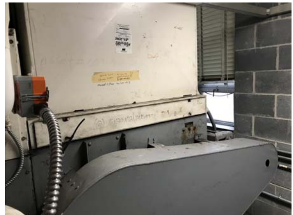
BREW060e 5/12/2021 Dual duct air handling unit Room C208
