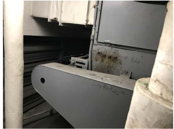
BREW067e 5/12/2021 Multizone air handling unit Room A245
