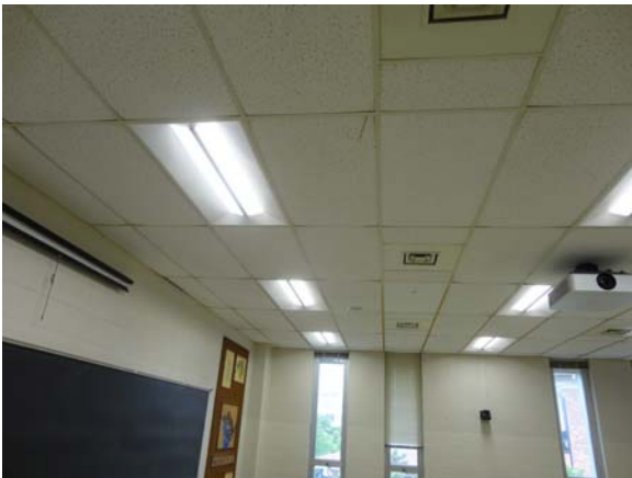
BREW051a 5/12/2021 Older acoustical ceiling with newer ceiling tiles D Wing, second floor classroom
