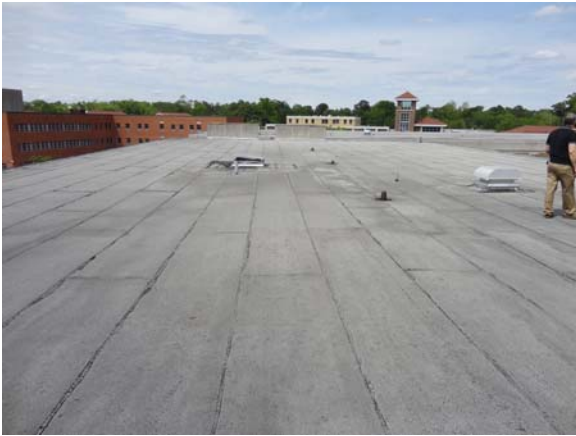
BREW004a 5/12/2021 Weathered built-up roof with cap sheet A Wing roof
