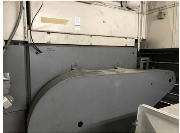
BREW049e 5/12/2021 Dual duct air handling unit Room D316
