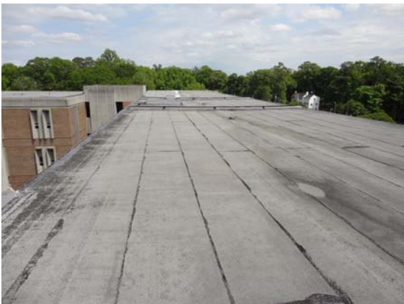
BREW003a 5/12/2021 Weathered built-up roof with cap sheet B Wing roof
