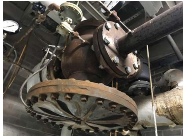
BREW032e 5/12/2021 Pressure reducing valve Room B109
