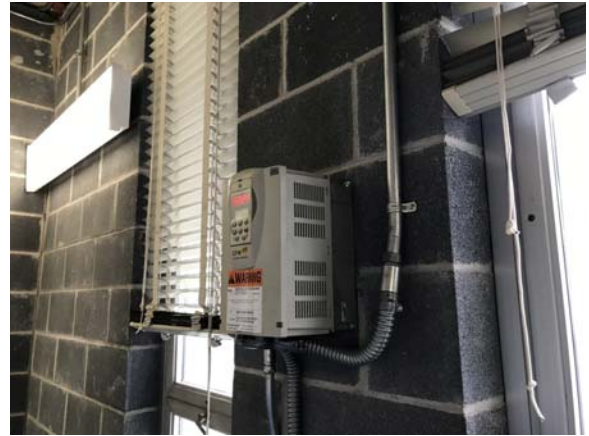
BREW058e 5/12/2021 VFD for air handling unit Room C309
