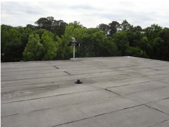
BREW012a 5/12/2021 No fall protection for the various rooftop speakers Main roof
