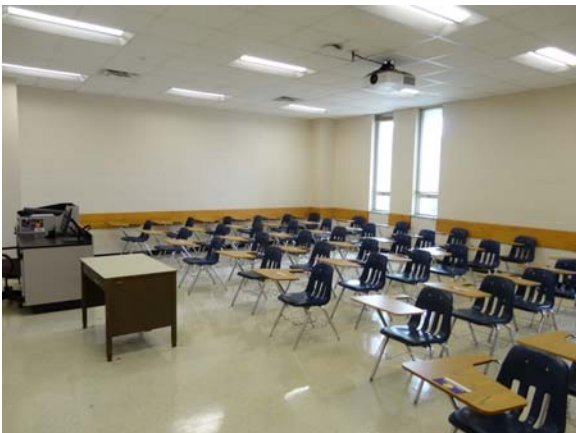
BREW024a 5/12/2021 Older vinyl floor tile and older acoustical ceiling B Wing, third floor classroom
