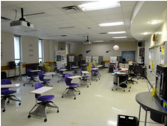
BREW044a 5/12/2021 Older vinyl flooring and acoustical ceiling D Wing, first floor classroom
