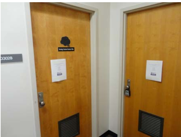
BREW057a 5/12/2021 Older interior doors with knob hardware D Wing, third floor office area
