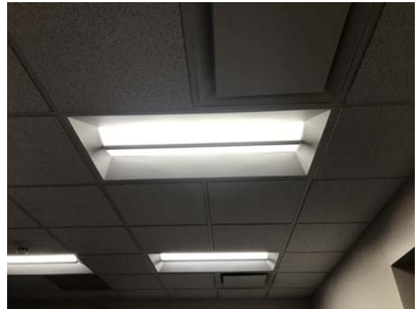
BREW044e 5/12/2021 Recessed LED lighting fixture Room D107
