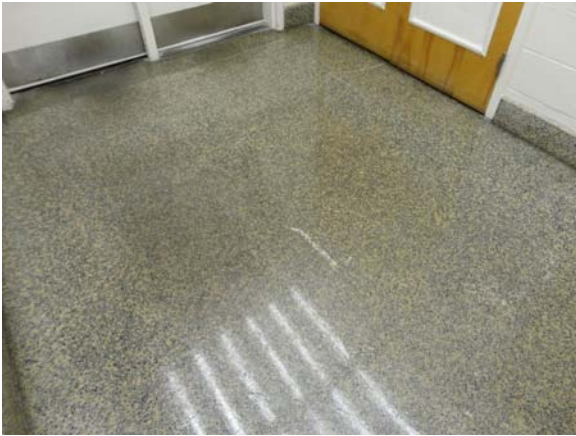
BREW052a 5/12/2021 Worn terrazzo flooring D Wing, third floor corridor
