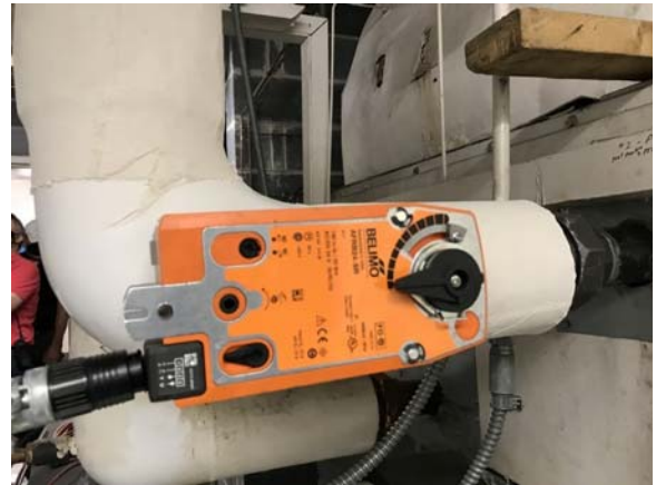
BREW059e 5/12/2021 DDC valve positioners Room C208
