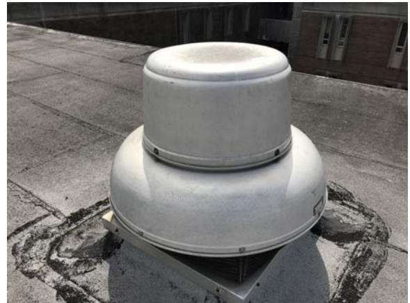
BREW005e 5/12/2021 Centrifugal rooftop exhaust fan Roof
