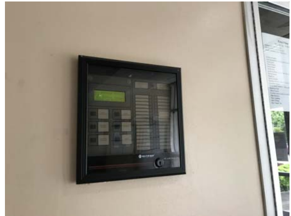
BREW071e 5/12/2021 Fire alarm annunciator panel A Wing, lobby
