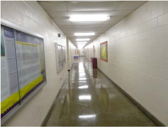
BREW049a 5/12/2021 Worn terrazzo, sagging acoustical ceiling, and painted CMU D Wing, second floor corridor
