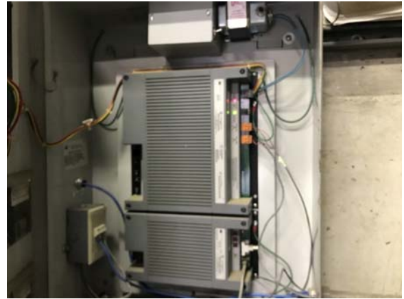
BREW025e 5/12/2021 HVAC field panel Room B109
