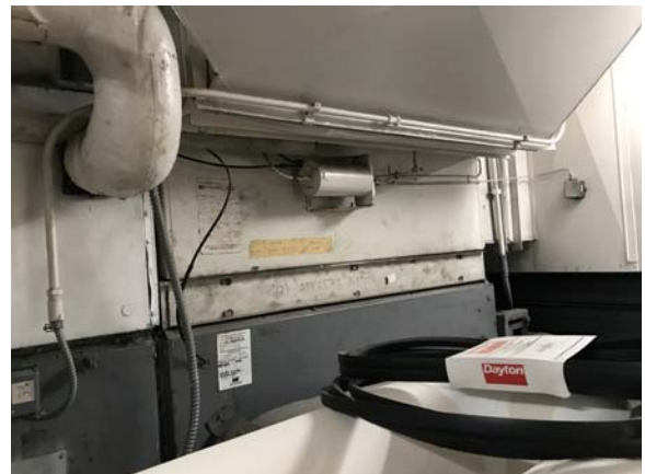
BREW045e 5/12/2021 Dual duct air handling unit Room D116
