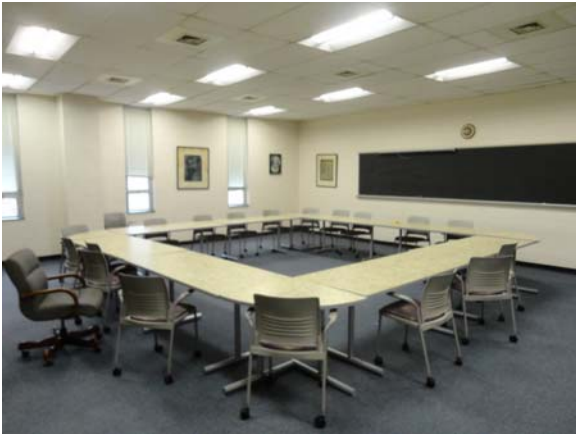
BREW055a 5/12/2021 Older carpeting and acoustical ceiling D Wing third floor classroom
