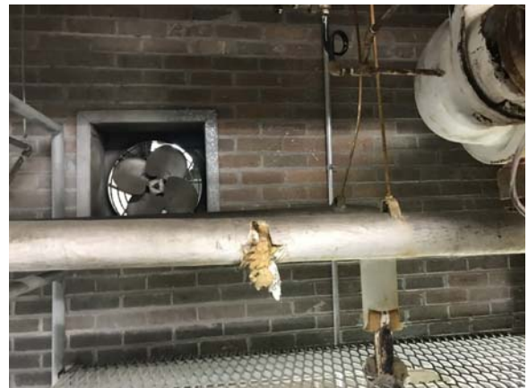
BREW033e 5/12/2021 Propeller exhaust fan Room B109
