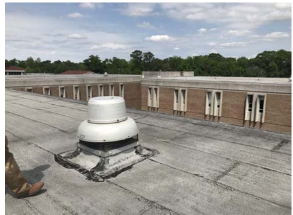
BREW003e 5/12/2021 Centrifugal rooftop exhaust fan Roof
