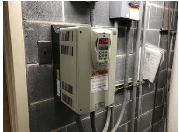
BREW051e 5/12/2021 VFD for air handling unit Room D316
