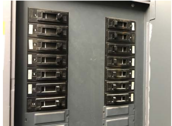
BREW007e 5/12/2021 Local panelboard Room B309
