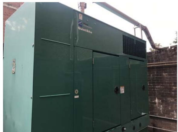
BREW021e 5/12/2021 Diesel-fired emergency generator B Wing site
