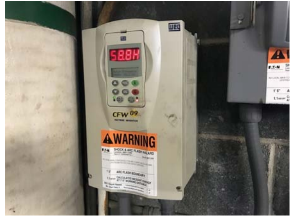
BREW017e 5/12/2021 VFD for air handling unit Room B209
