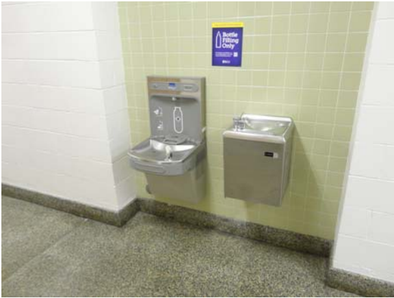
BREW034a 5/12/2021 New and old single-level water fountains B Wing, first floor corridor
