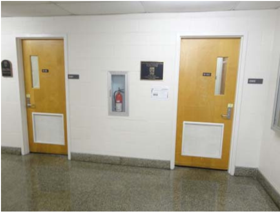
BREW058a 5/12/2021 Older nonrated doors with transfer louvers D Wing, third floor corridor
