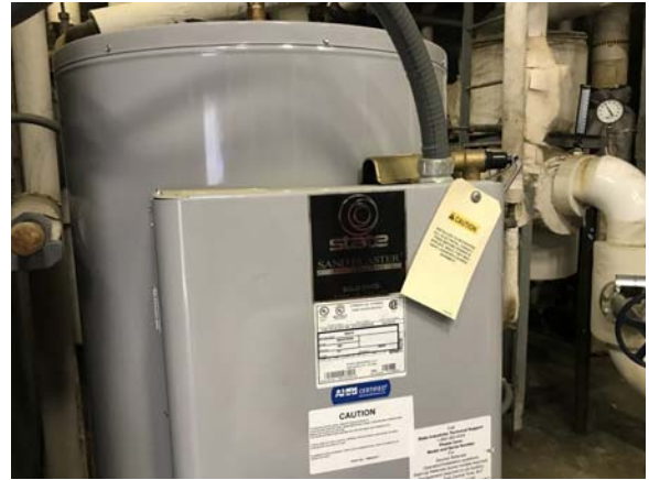
BREW028e 5/12/2021 Electric water heater Room B109
