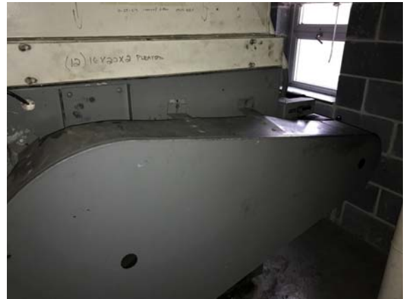
BREW056e 5/12/2021 Dual duct air handling unit Room C309
