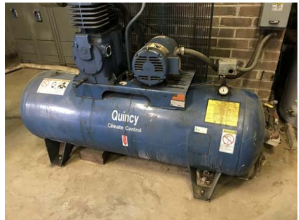
BREW027e 5/12/2021 Controls air compressor Room B109
