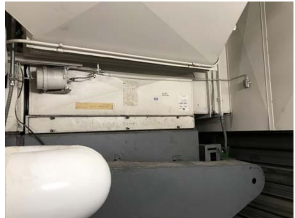
BREW047e 5/12/2021 Dual duct air handling unit Room D219
