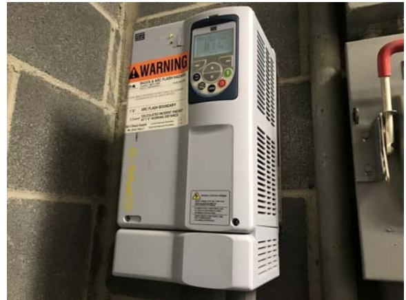
BREW068e 5/12/2021 VFD for air handling unit Room A245
