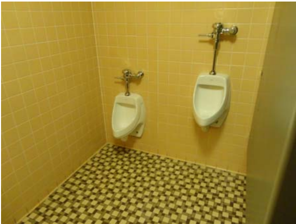
BREW032a 5/12/2021 Accessible wall-hung urinals B Wing, first floor men's restroom
