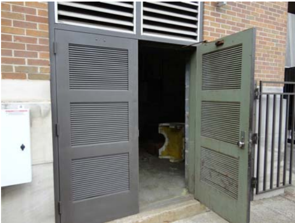
BREW038a 5/12/2021 Aging original hollow-metal service doors B Wing, first floor mechanical area
