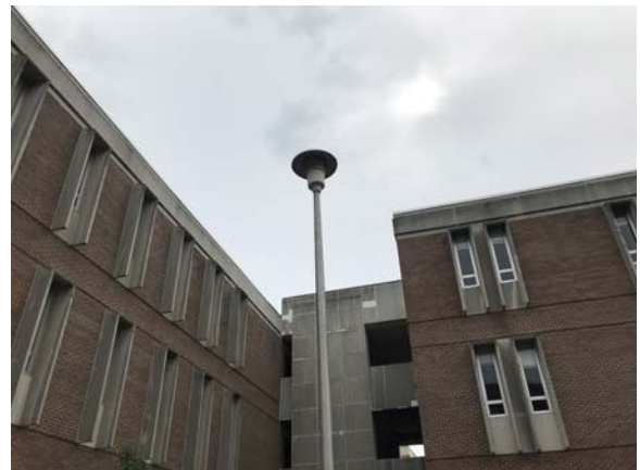
BREW072e 5/12/2021 Pole-mounted LED lighting fixture Courtyard
