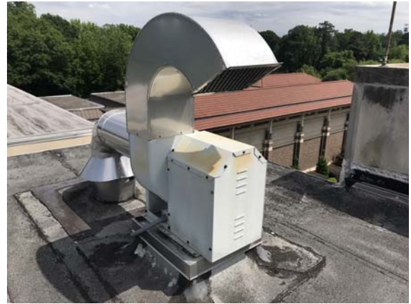
BREW004e 5/12/2021 Utility-style exhaust fan Roof
