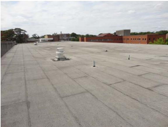
BREW008a 5/12/2021 Weathered built-up roof with cap sheet D Wing roof
