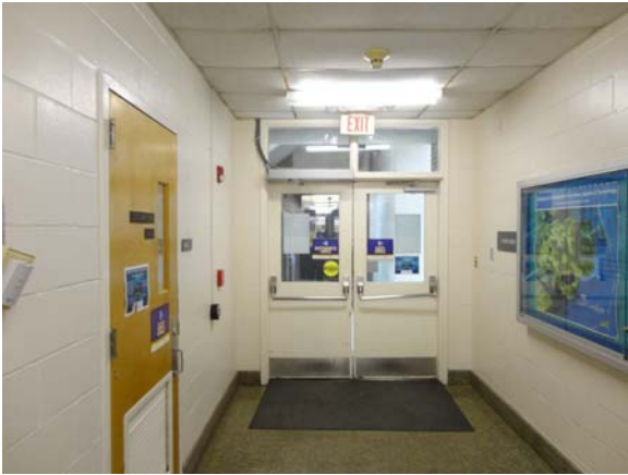
BREW037a 5/12/2021 Older exterior doors with panic hardware B Wing, first floor corridor
