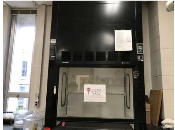
BREW052e 5/12/2021 Fume hood Room D211
