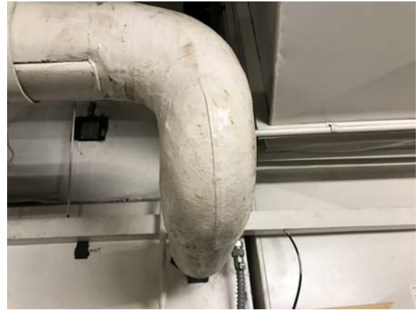
BREW050e 5/12/2021 Potential asbestos insulation on mechanical piping Room D316
