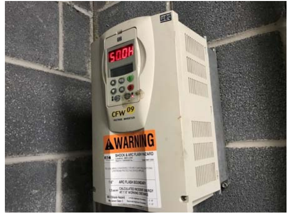
BREW064e 5/12/2021 VFD for air handling unit Room A445
