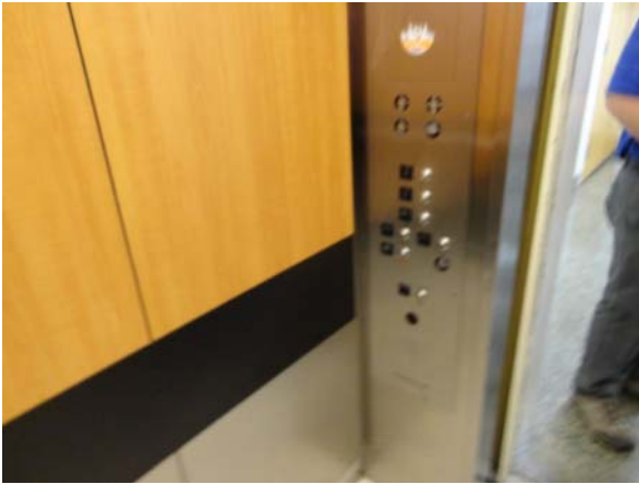
BREW001a 5/12/2021 Accessible elevator control panel B Wing, passenger elevator
