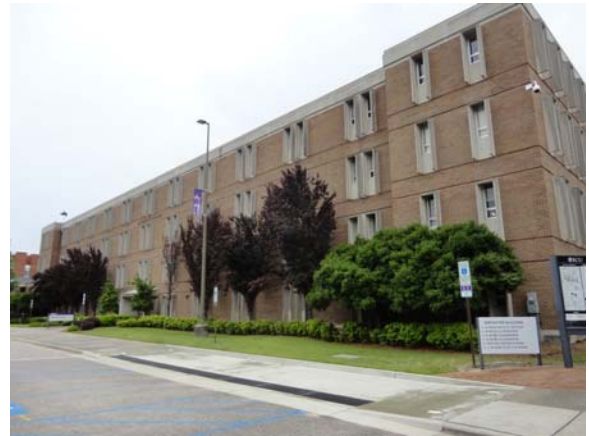
BREW088a 5/12/2021 Brick facade and stained cut stone facades South elevation of A Wing
