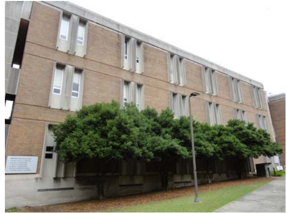
BREW086a 5/12/2021 Brick facade and stained cut stone facades East elevation of C Wing
