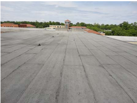
BREW006a 5/12/2021 Weathered built-up roof with cap sheet C Wing roof
