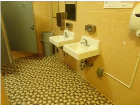
BREW033a 5/12/2021 Older wall-hung lavatories B Wing, first floor men's restroom
