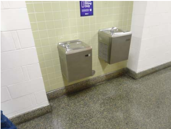
BREW029a 5/12/2021 Older two-level water fountain B Wing, second floor corridor
