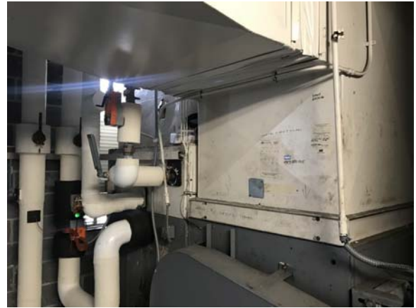
BREW016e 5/12/2021 Dual duct air handling unit Room B209
