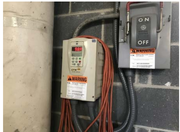
BREW009e 5/12/2021 VFD for air handling unit Room B309
