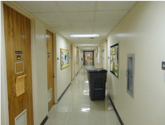
BREW071a 5/12/2021 Older vinyl flooring and acoustical ceiling A Wing, fourth floor corridor
