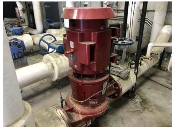
BREW024e 5/12/2021 Heating hot water pump Room B109
