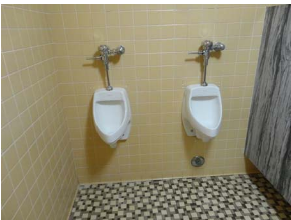
BREW018a 5/12/2021 Wall-hung urinals B Wing, third floor men's restroom
