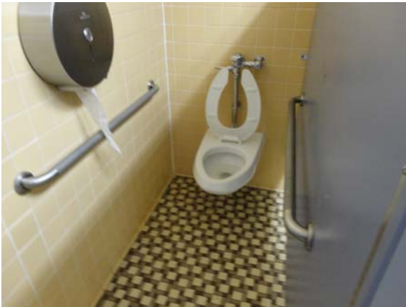
BREW047a 5/12/2021 Older, partially accessible toilet stall D Wing, first floor men's restroom
