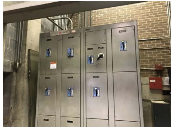
BREW035e 5/12/2021 Main switchboard Room B109
