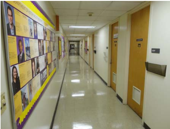
BREW075a 5/12/2021 Older vinyl flooring and acoustical ceiling A Wing, third floor corridor
