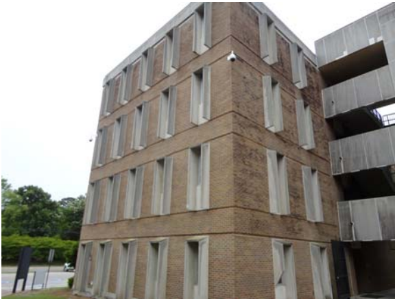
BREW087a 5/12/2021 Some upper staining and lower broken stone solar fin East end of A Wing
