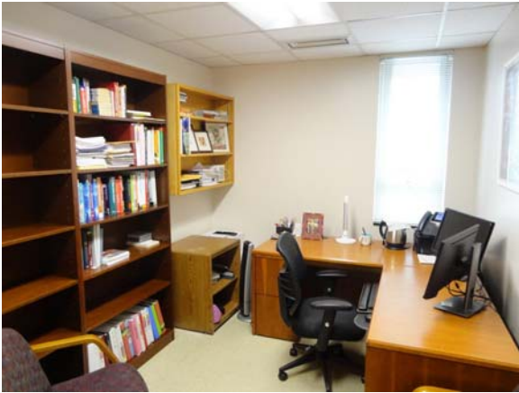
BREW073a 5/12/2021 Older vinyl flooring and acoustical ceiling A Wing, third floor office
