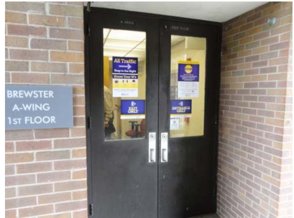
BREW076a 5/12/2021 Older narrow double two-foot, six-inch entry doors A Wing, first floor entry
