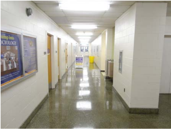
BREW016a 5/12/2021 Worn terrazzo, sagging acoustical ceiling, and painted CMU B Wing, third floor corridor
