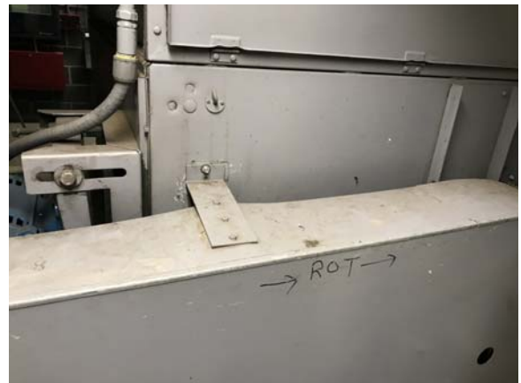
BREW069e 5/12/2021 Multizone air handling unit Room A139
