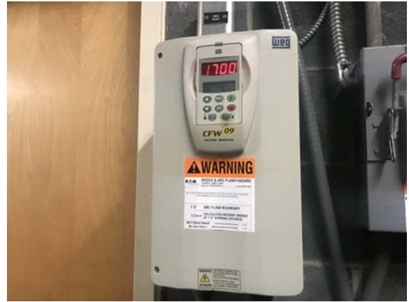
BREW046e 5/12/2021 VFD for air handling unit Room D116
