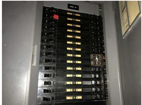
RAWL017e 5/10/2021 Local panelboard Classroom
