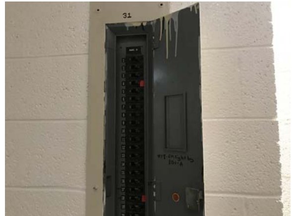
RAWL011e 5/10/2021 Local panelboard Third floor corridor
