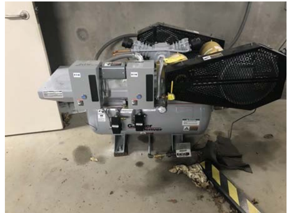
RAWL041e 5/10/2021 Controls air compressor Room 147
