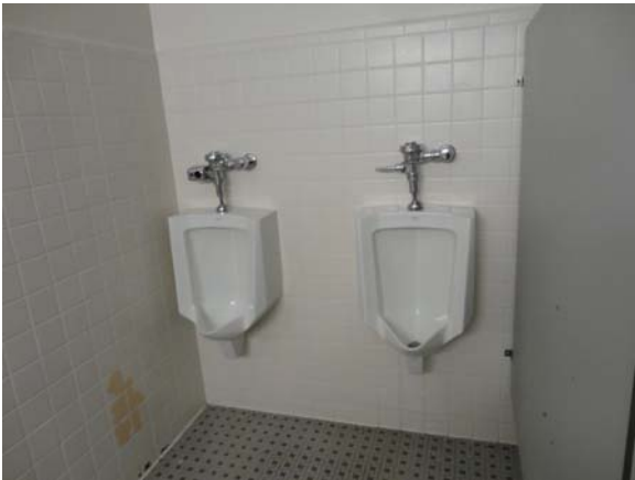
RAWL032a 5/10/2021 Wall-mounted urinals and older ceramic wall and floor tile First floor men's restroom
