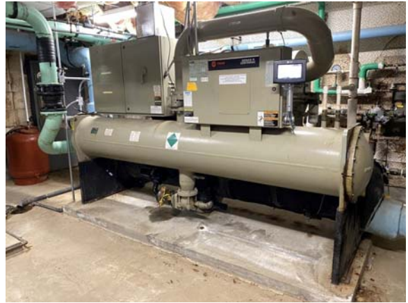
RAWL001e 5/10/2021 Water-cooled centrifugal chiller Room 12A
