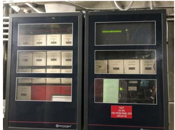
RAWL038e 5/10/2021 Main fire alarm panel Room 147
