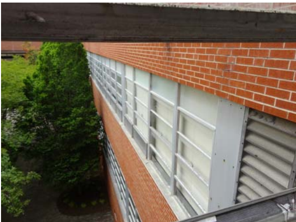
RAWL018a 5/10/2021 Aging original upper glazing Upper elevation
