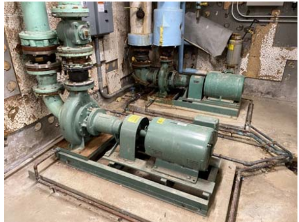
RAWL002e 5/10/2021 Chilled water and condenser water pumps Room 12A
