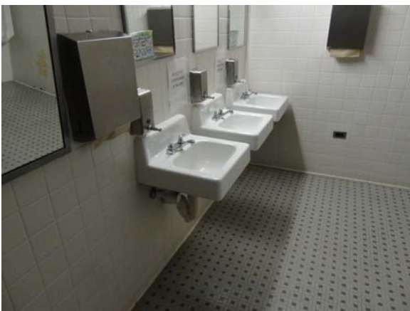
RAWL033a 5/10/2021 Three standard wall lavatories First floor men's restroom
