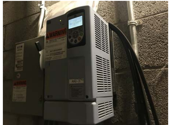
RAWL020e 5/10/2021 VFD for AHU-003 Room 246
