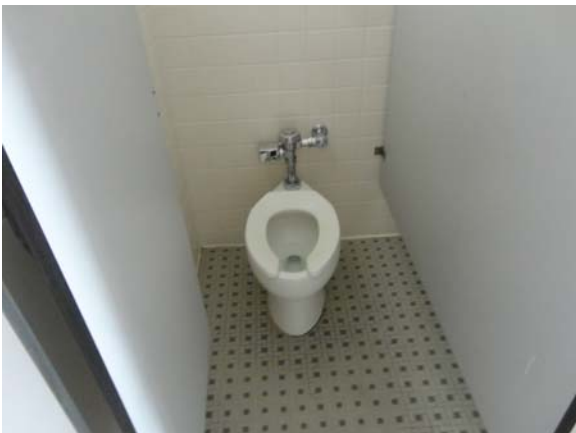
RAWL024a 5/10/2021 Standard tankless toilet Second floor women's restroom
