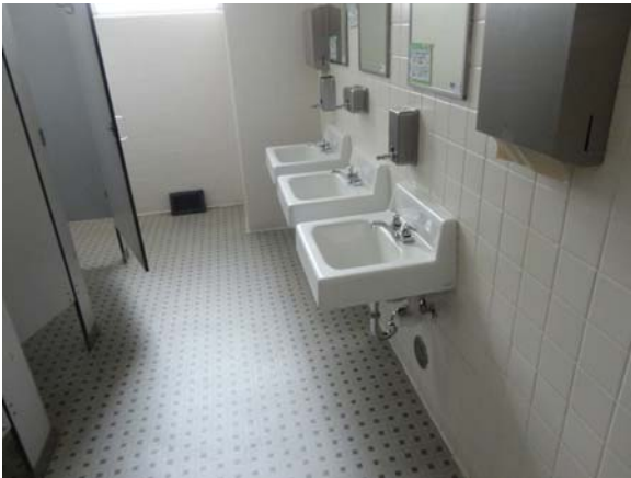
RAWL023a 5/10/2021 Standard wall-mounted lavatories Second floor women's restroom
