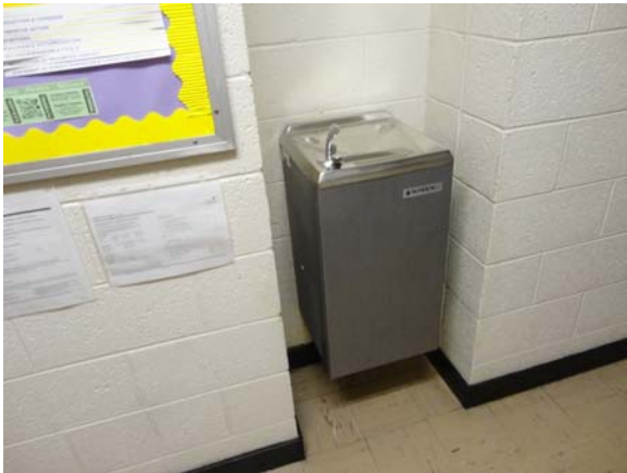
RAWL045a 5/10/2021 Aging single-level water fountain Annex basement corridor
