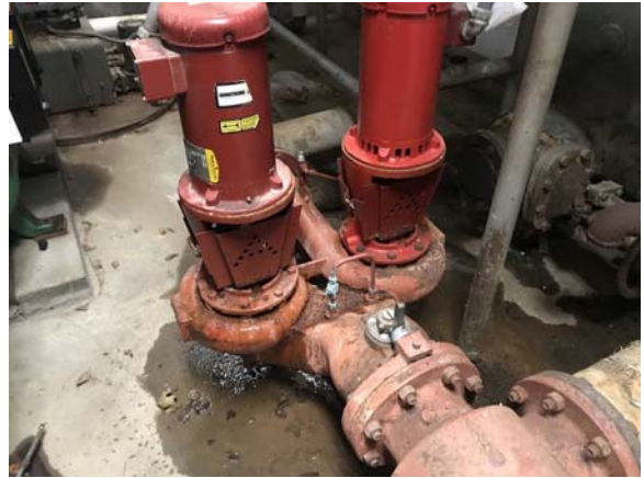
RAWL034e 5/10/2021 Inline heating hot water pumps Room 147
