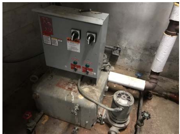
RAWL036e 5/10/2021 Condensate receiver Room 147
