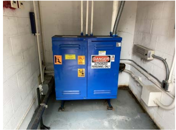
RAWL007e 5/10/2021 Hydraulic elevator controls Room 101
