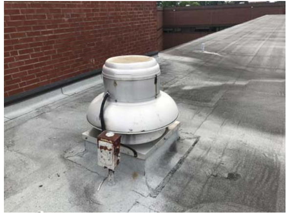
RAWL013e 5/10/2021 Centrifugal rooftop exhaust fan Roof
