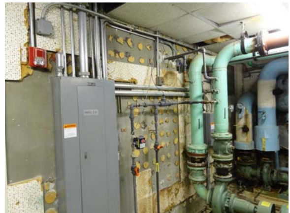
RAWL066a 5/10/2021 Deteriorated adhesive wall tile suspected to contain asbestos Basement mechanical roof
