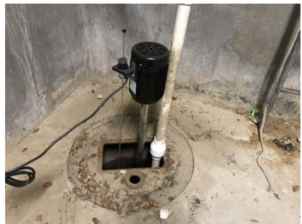
RAWL033e 5/10/2021 Sump pump Room 147
