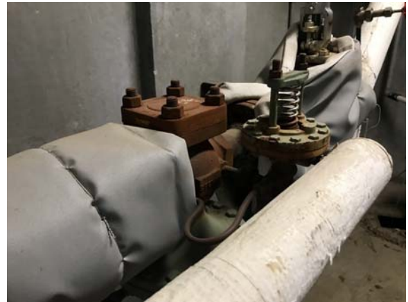
RAWL032e 5/10/2021 Pressure reducing valve Room 147
