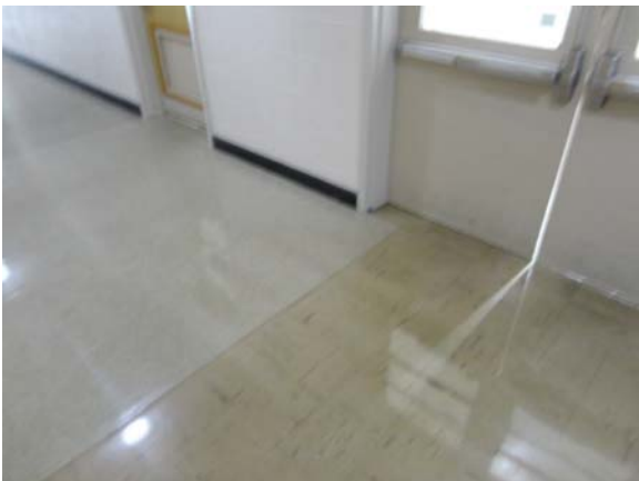
RAWL021a 5/10/2021 Dissimilar vinyl floor tile repairs Second floor corridor
