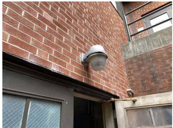
RAWL003e 5/10/2021 HID sconce lighting fixture Exterior entrance
