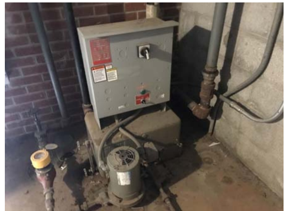
RAWL030e 5/10/2021 Condensate receiver Room 009
