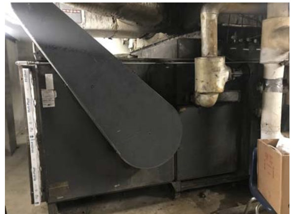
RAWL039e 5/10/2021 Air handling unit AHU-001 Room 147
