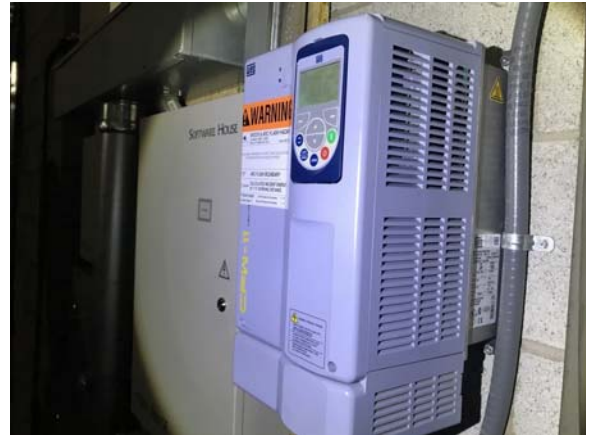
RAWL025e 5/10/2021 VFD for AHU-002 Room 145
