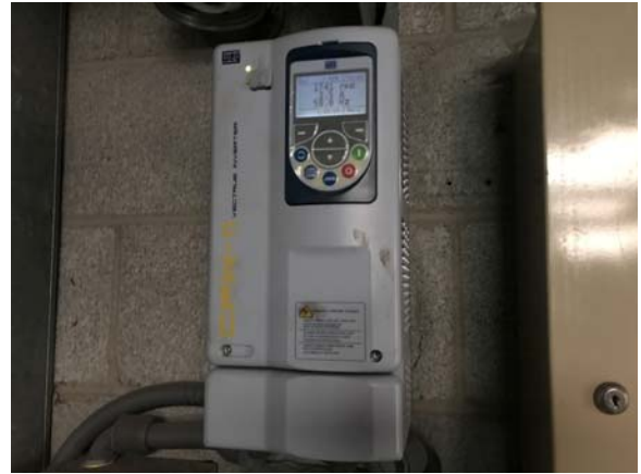
RAWL028e 5/10/2021 VFD for AHU-005 Room 247
