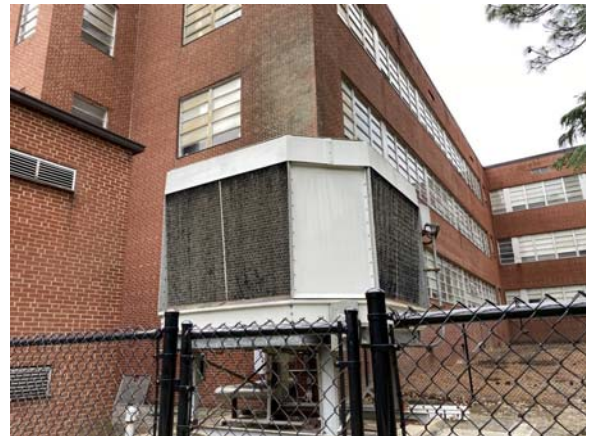
RAWL006e 5/10/2021 Cooling tower Exterior
