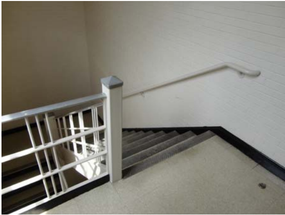
RAWL004a 5/10/2021 Accessible wall rail but wide picket spacing on inner railing Third floor, stair tower
