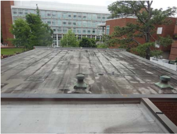
RAWL028a 5/10/2021 Weathered built-up roof South annex roof
