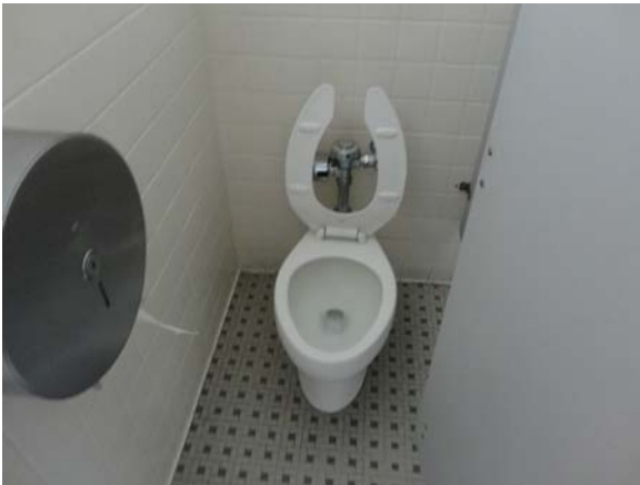
RAWL017a 5/10/2021 Standard tankless toilet Third floor men's restroom
