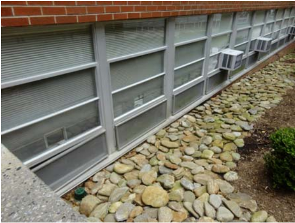
RAWL049a 5/10/2021 Exterior window too close to grade Annex
