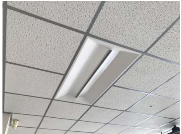
RAWL014e 5/10/2021 Recessed lay-in LED lighting Room 339
