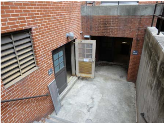
RAWL065a 5/10/2021 Aging hollow metal service doors in areaway Southwest areaway
