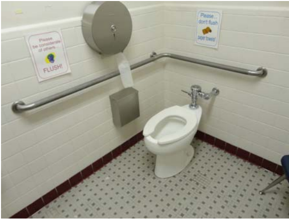
RAWL010a 5/10/2021 Accessible tankless toilet Third floor all-gender restroom
