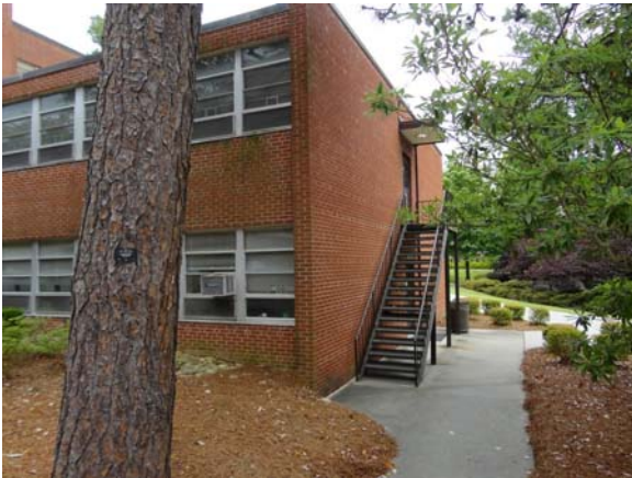
RAWL051a 5/10/2021 Exterior metal stair with open risers South end of south annex wing
