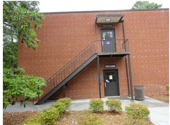
RAWL052a 5/10/2021 Hollow metal exterior egress doors South end of south annex wing
