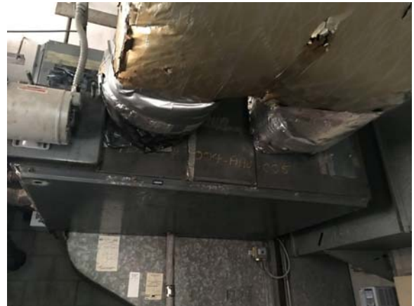
RAWL026e 5/10/2021 Fan coil unit AHU-005 Room 247
