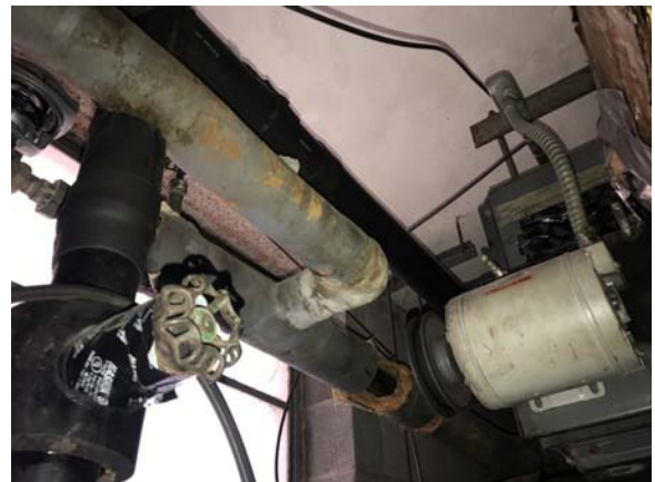
RAWL027e 5/10/2021 Potential asbestos insulation on mechanical piping Room 247
