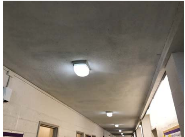
RAWL010e 5/10/2021 Ceiling-mounted sconce lighting fixture Third floor corridor
