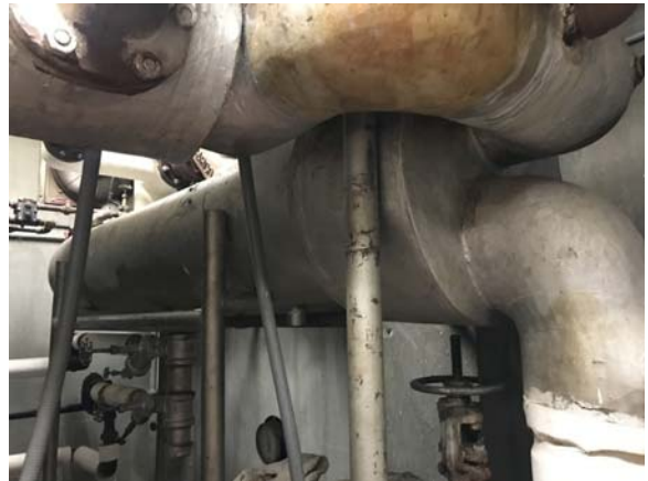
RAWL035e 5/10/2021 Heating hot water shell-and-tube heat exchanger Room 147
