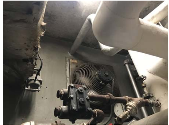
RAWL037e 5/10/2021 Propeller exhaust fan Room 147
