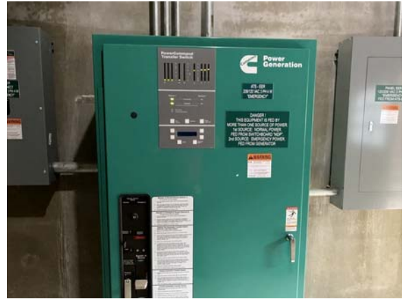
RAWL005e 5/10/2021 Automatic transfer switch Room 146
