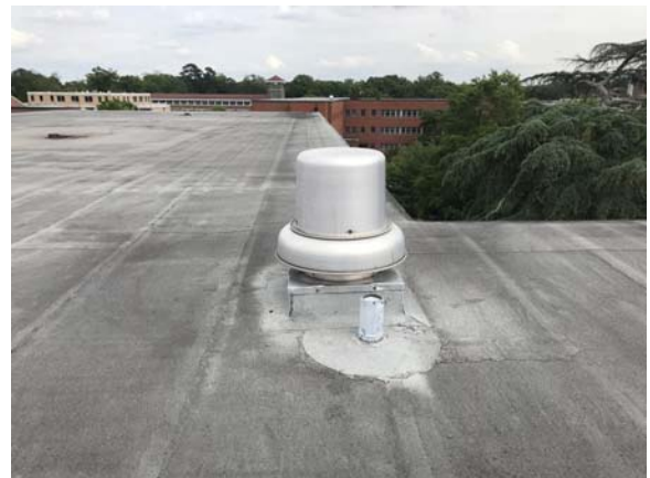
RAWL012e 5/10/2021 Centrifugal rooftop exhaust fan Roof
