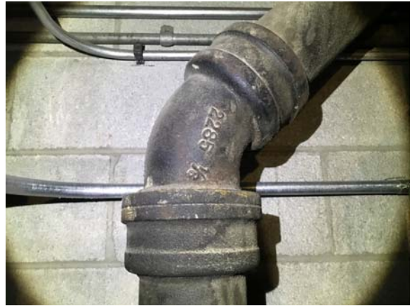
RAWL022e 5/10/2021 Cast-iron drain piping with bell-and-spigot connection Room 246
