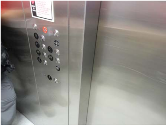
RAWL001a 5/10/2021 Accessible elevator control panel East elevator tower addition
