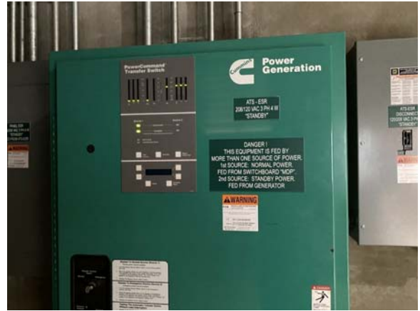
RAWL004e 5/10/2021 Automatic transfer switch Room 146
