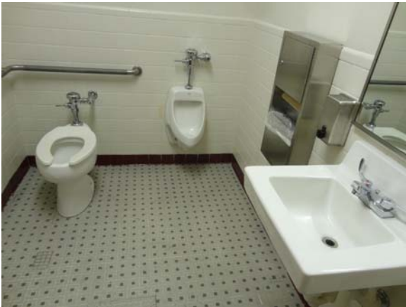
RAWL035a 5/10/2021 Three-fixture accessible restroom, noting older ceramic tile First floor all-gender restroom
