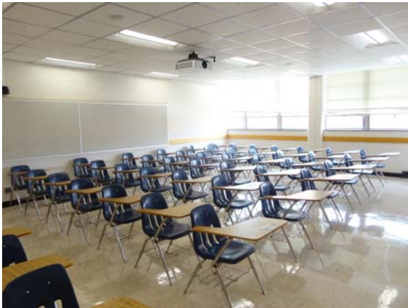
RAWL008a 5/10/2021 Older vinyl composite floor tile and acoustical ceiling Third floor classroom
