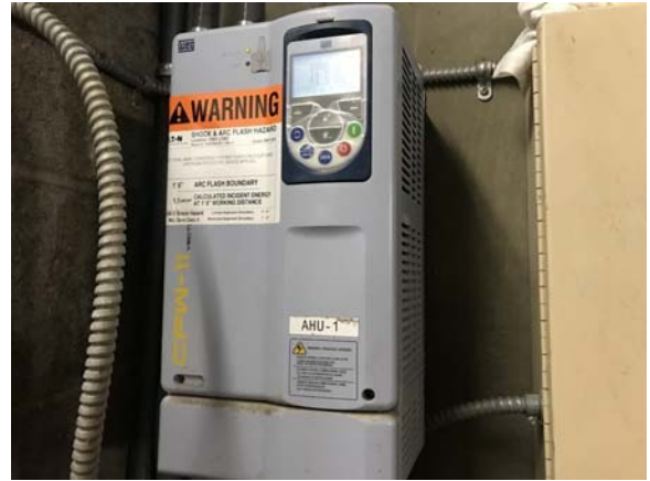
RAWL040e 5/10/2021 VFD for AHU-001 Room 147
