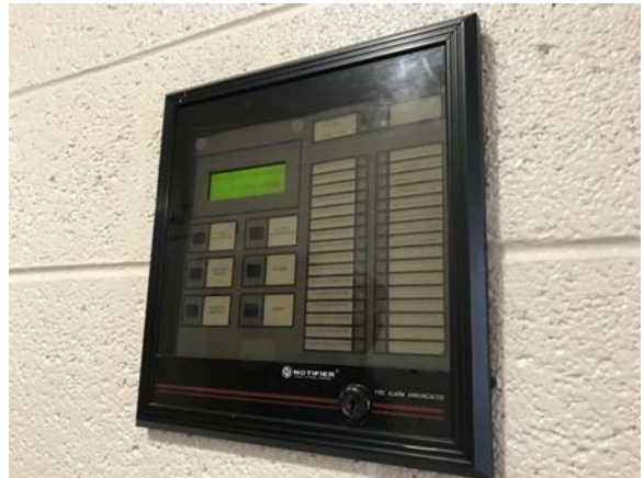
RAWL023e 5/10/2021 Fire alarm annunciator panel First floor lobby
