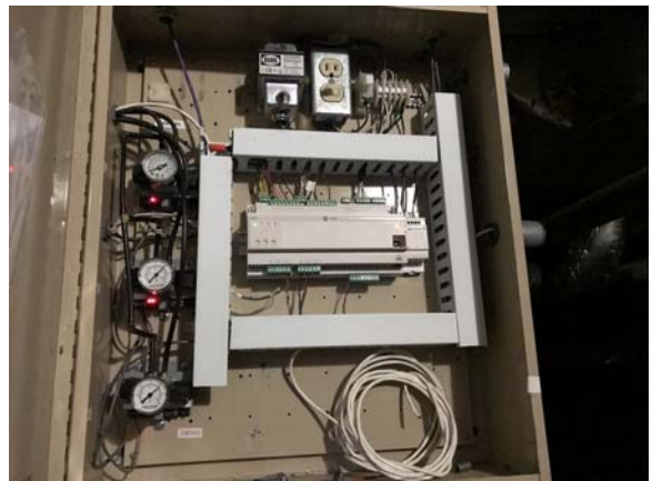
RAWL018e 5/10/2021 HVAC field panel Room 246
