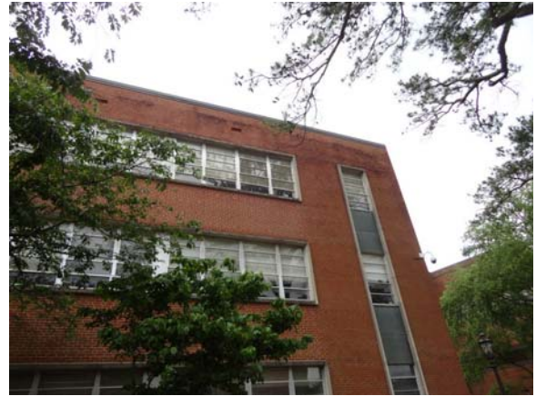
RAWL062a 5/10/2021 Light staining on upper brick Upper north elevation
