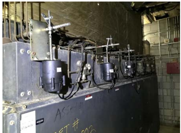
RAWL024e 5/10/2021 Air handling unit AHU-002 Room 145
