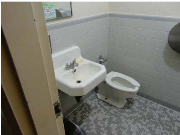
RAWL047a 5/10/2021 Aging standard fixturing Annex basement restroom
