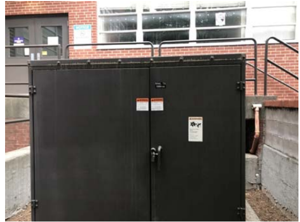
RAWL031e 5/10/2021 Oil-filled transformer Exterior
