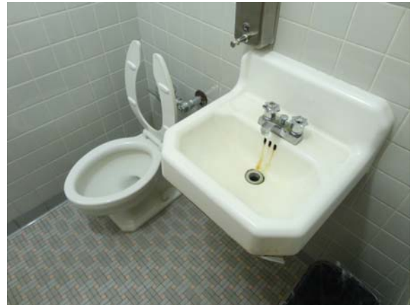
RAWL046a 5/10/2021 Aging standard fixturing Annex basement restroom
