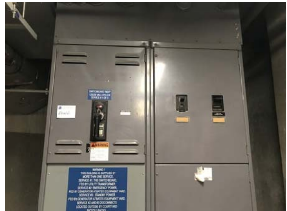
RAWL042e 5/10/2021 Main switchboard Room 147
