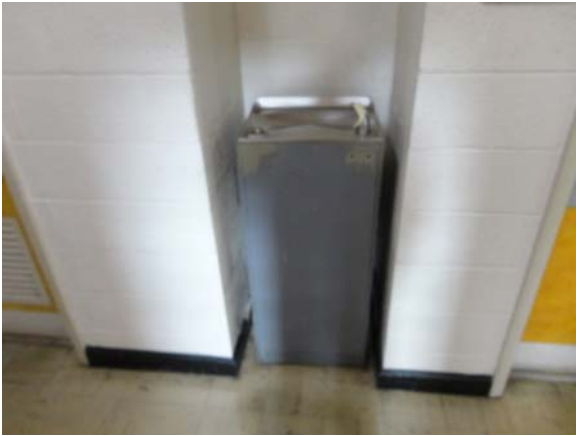
RAWL022a 5/10/2021 Aging freestanding water fountain Second floor corridor
