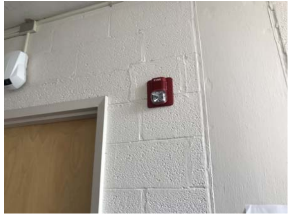
RAWL016e 5/10/2021 Horn strobe fire alarm device Third floor corridor
