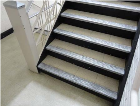
RAWL019a 5/10/2021 Loose metal stair nosing and aging vinyl tile treads Second floor, stair tower
