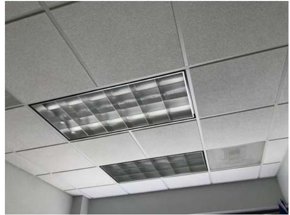
RIVW004e 5/12/2021 Open-cell grid recessed, lay-in T8 lighting fixtures Room RW-338
