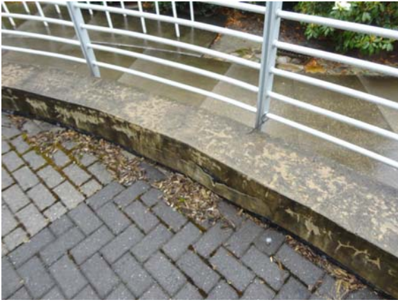
RIVW046a 5/12/2021 Spalling finish on plaza wall South plaza
