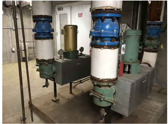
RIVW013e 5/12/2021 Heating hot water pumps Room RW-006
