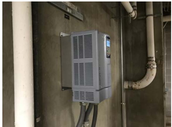
RIVW015e 5/12/2021 VFD for heating hot water pump Room RW-006
