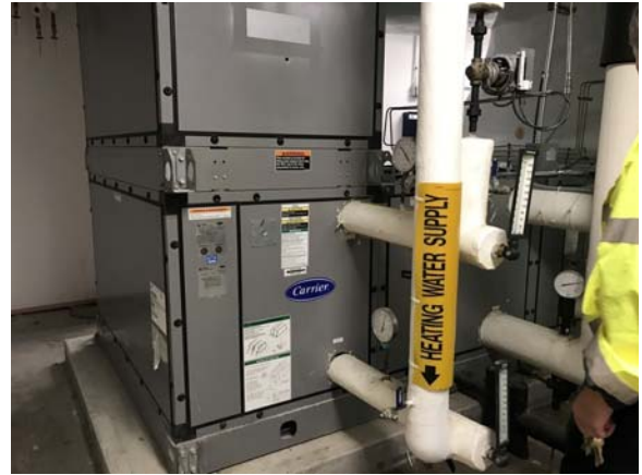
RIVW025e 5/12/2021 Air handling unit AHU-001 Room RW-118
