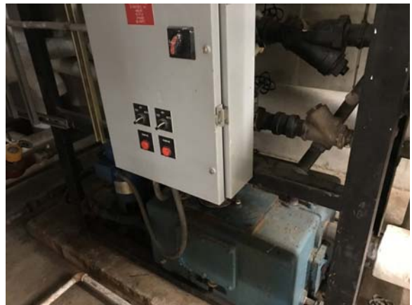
RIVW018e 5/12/2021 Condensate receiver Room RW-006
