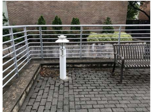
RIVW032e 5/12/2021 Bollard lighting fixture Site
