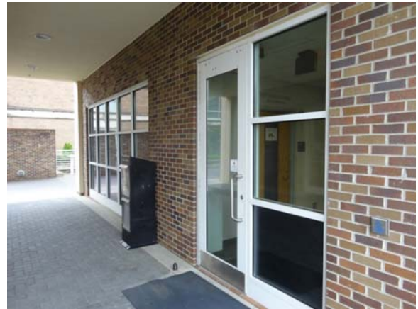
RIVW043a 5/12/2021 Power door assist on breezeway doors South breezeway
