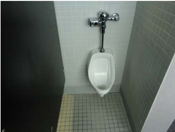
RIVW011a 5/12/2021 Wall-hung urinal Third floor, men's restroom
