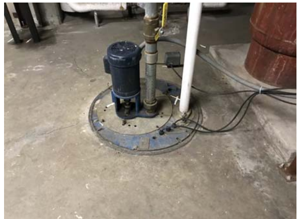
RIVW021e 5/12/2021 Sump pump Room RW-006
