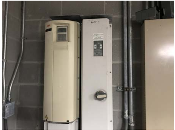
RIVW016e 5/12/2021 VFD for chilled water pump Room RW-006
