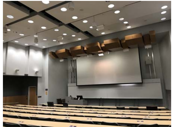
RIVW029e 5/12/2021 Recessed can lighting Auditorium RW-105A
