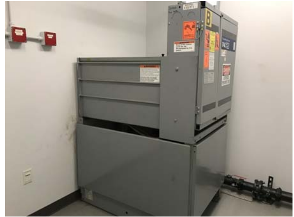
RIVW028e 5/12/2021 Hydraulic elevator controls Room RW-103
