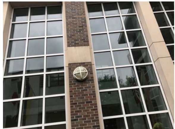
RIVW030e 5/12/2021 CFL sconce lighting fixture Exterior
