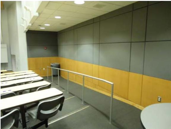
RIVW032a 5/12/2021 No outer handrail at side aisle ramp First floor, auditorium
