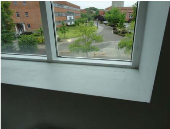
RIVW029a 5/12/2021 Minor window sill damage due to condensation Second floor window detail
