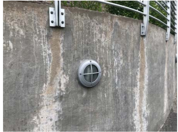
RIVW031e 5/12/2021 CFL sconce lighting fixture Exterior
