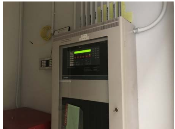
RIVW024e 5/12/2021 Main fire alarm panel Room RW-119
