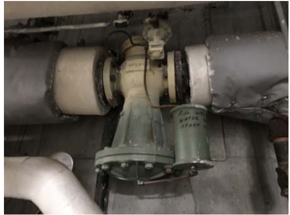
RIVW019e 5/12/2021 Pressure reducing valve Room RW-006
