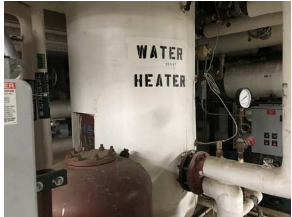
RIVW020e 5/12/2021 Domestic hot water heat exchanger Room RW-006
