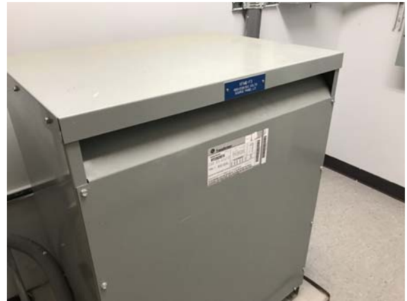
RIVW005e 5/12/2021 Secondary step-down transformer Room RW-321
