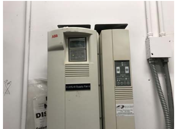
RIVW026e 5/12/2021 VFD for AHU-001 supply fan Room RW-118
