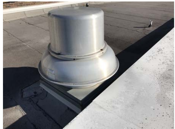
RIVW033e 5/12/2021 Centrifugal rooftop exhaust fan Roof
