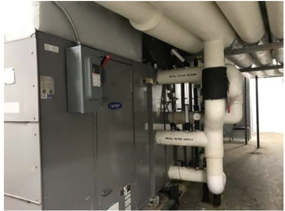
RIVW007e 5/12/2021 Air handling unit AHU-002 Room RW-222
