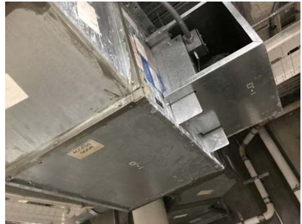
RIVW023e 5/12/2021 Inline centrifugal exhaust fan Room RW-006
