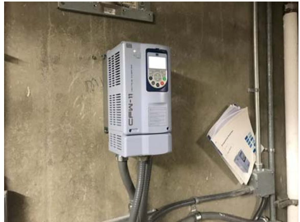
RIVW014e 5/12/2021 VFD for heating hot water pump Room RW-006
