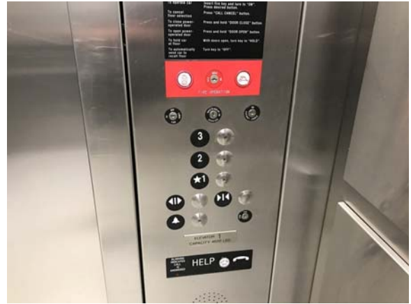
RIVW001e 5/12/2021 Elevator control panel Elevator
