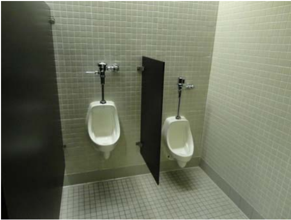
RIVW025a 5/12/2021 Wall-hung urinals Second floor, men's restroom
