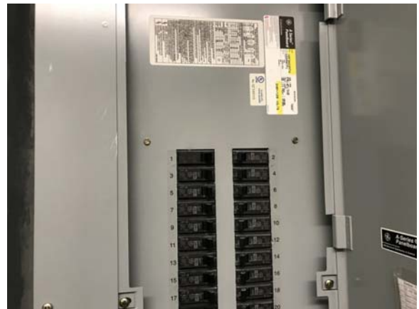
RIVW006e 5/12/2021 Local panelboard Room RW-321
