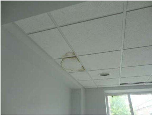
RIVW022a 5/12/2021 Ceiling tile stains due to possible roof leak Second floor link to Rivers Building
