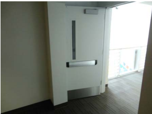
RIVW021a 5/12/2021 Corridor isolation doors on magnetic hold backs Second floor, central east corridor
