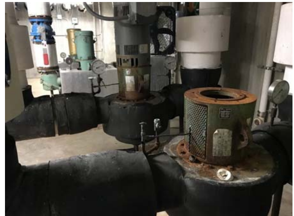
RIVW012e 5/12/2021 Chilled water pumps Room RW-006
