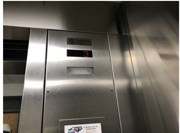
RIVW002e 5/12/2021 Elevator interior Elevator
