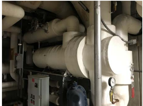
RIVW017e 5/12/2021 Heating hot water shell-and-tube heat exchanger Room RW-006
