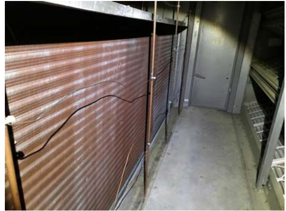
RIVW010e 5/12/2021 Interior coils of AHU-002 Room RW-222
