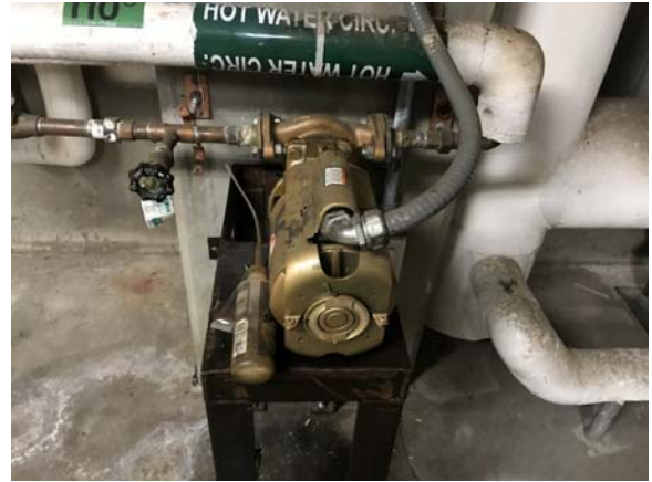
RIVW022e 5/12/2021 Domestic hot water pump Room RW-006
