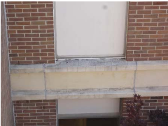
RIVE006a 5/13/2021 Some stress cracks in precast banding Upper facade exterior precast
