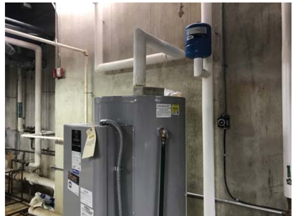
RIVE045e 5/13/2021 Residential electric water heater Room 03
