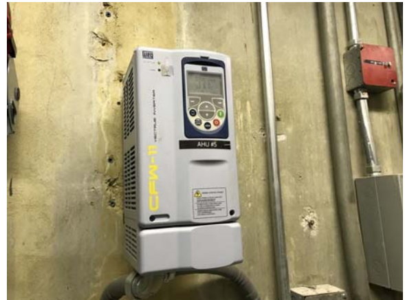
RIVE050e 5/13/2021 VFD for AHU-005 Room 03
