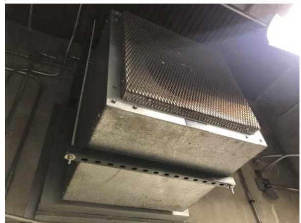
RIVE051e 5/13/2021 Propeller exhaust fan Room 03
