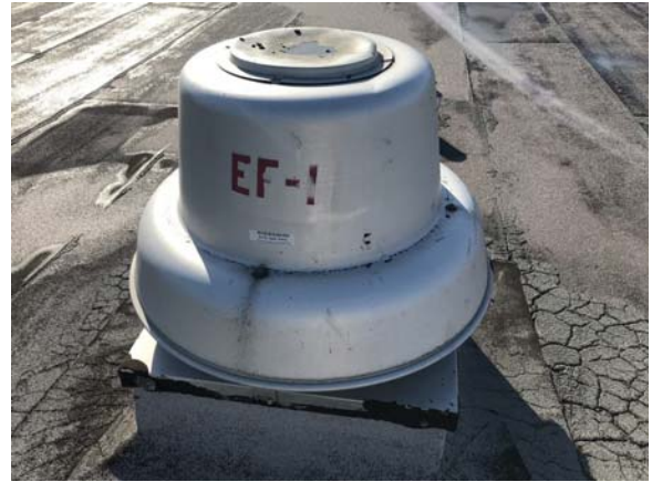
RIVE001e 5/13/2021 Centrifugal rooftop exhaust fan Roof
