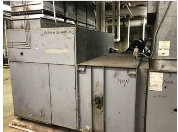
RIVE043e 5/13/2021 Air handling unit AHU-005 Room 03
