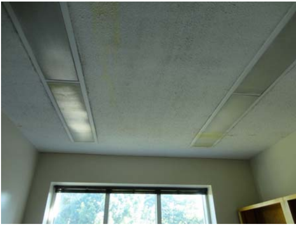
RIVE041a 5/13/2021 Stained textured ceiling Second floor, office
