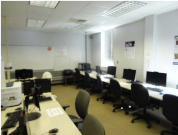
RIVE031a 5/13/2021 Older broadloom carpeting and acoustical ceiling Second floor, computer lab
