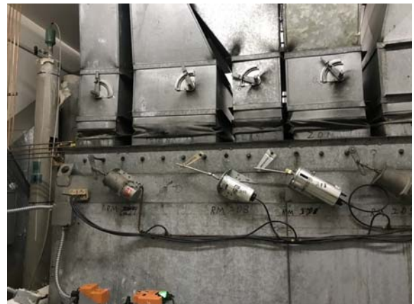
RIVE021e 5/13/2021 Air handling unit AHU-005 Room 214
