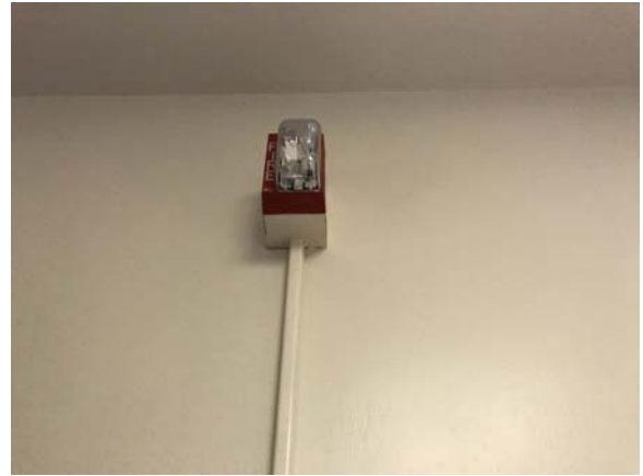
RIVE014e 5/13/2021 Horn with strobe fire alarm device Second floor corridor
