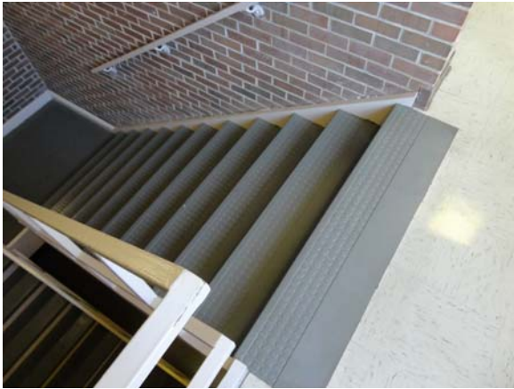
RIVE034a 5/13/2021 Rubber stair treads in average condition Second floor, central stair tower
