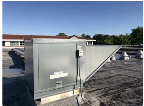
RIVE006e 5/13/2021 Fresh air makeup air handling unit Roof
