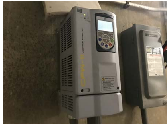
RIVE040e 5/13/2021 VFD for AHU-001 Room 02
