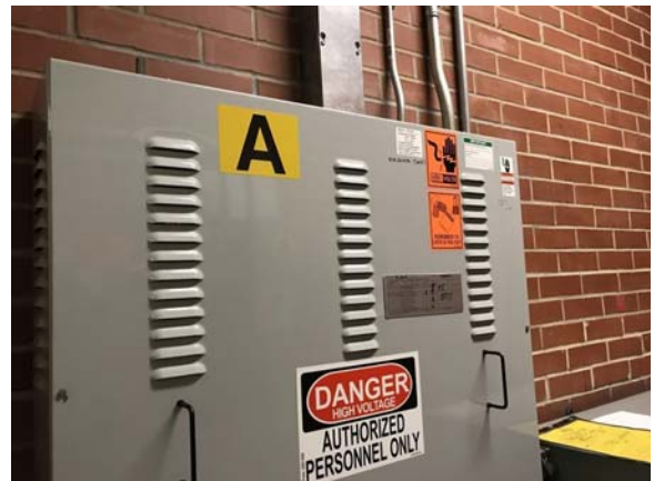
RIVE036e 5/13/2021 Elevator A controls Room 111
