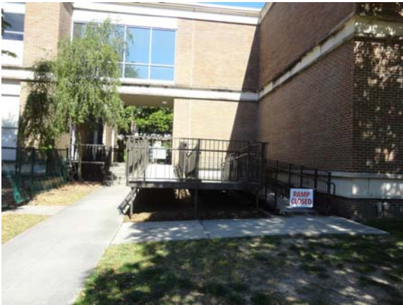
RIVE081a 5/13/2021 Rusted out pedestrian entry ramp Southeast elevation
