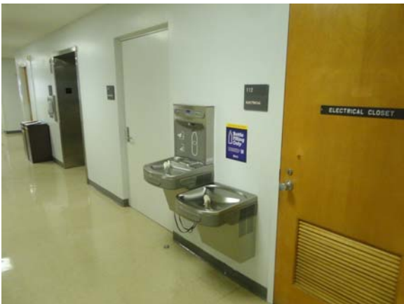
RIVE066a 5/13/2021 Newer dual-level water fountain First floor, north corridor
