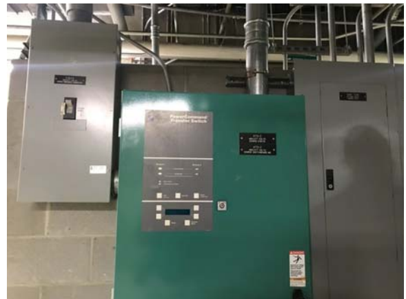
RIVE048e 5/13/2021 Automatic transfer switch Room 03
