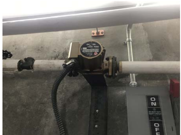
RIVE065e 5/13/2021 Domestic hot water circulation pump Room 05
