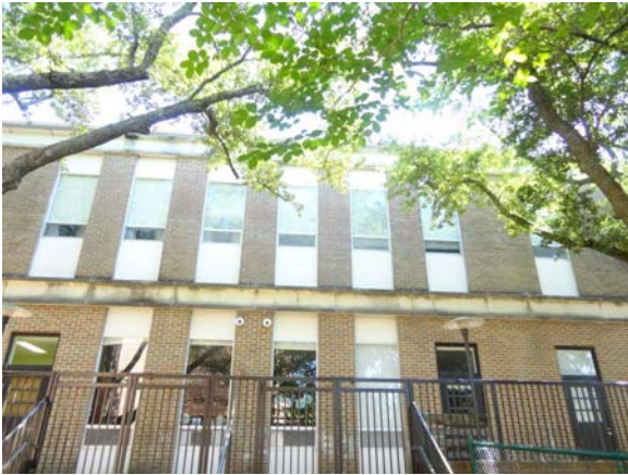
RIVE085a 5/13/2021 Staining visible on upper banding South elevation
