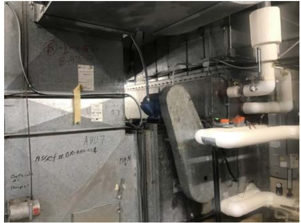
RIVE061e 5/13/2021 Air handling unit AHU-007 Room 05
