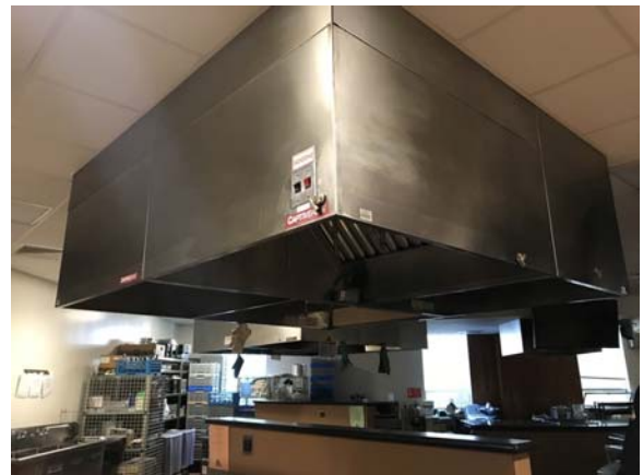
RIVE024e 5/13/2021 Commercial kitchen hood Room 158
