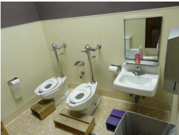
RIVE045a 5/13/2021 Two children's water closets and one wall-hung lavatory First floor, south daycare area
