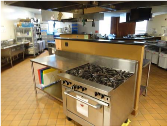
RIVE058a 5/13/2021 Quarry tile floor and staged cooking equipment First floor, teaching kitchen
