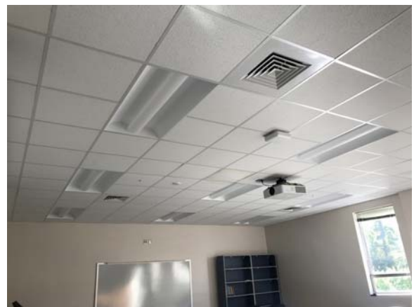
RIVE015e 5/13/2021 Recessed, lay-in LED lighting fixtures Room 260
