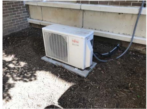
RIVE055e 5/13/2021 Ductless split condensing unit Site
