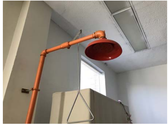
RIVE019e 5/13/2021 Emergency shower Room 258
