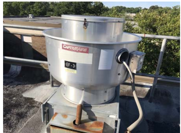
RIVE009e 5/13/2021 Kitchen exhaust fan Roof
