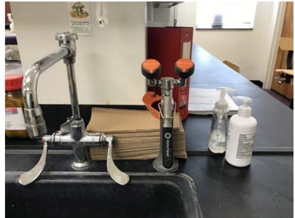
RIVE035e 5/13/2021 Emergency eyewash station Room 110C
