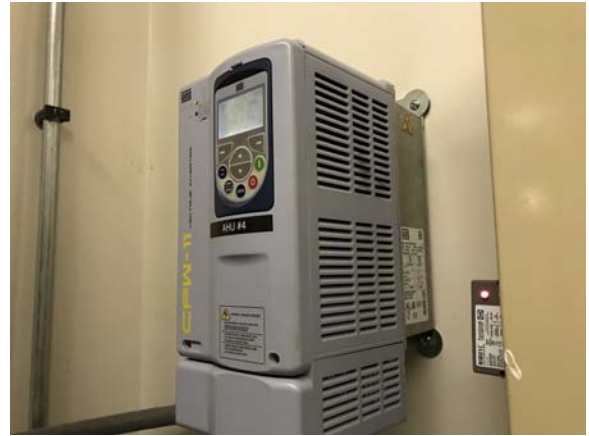
RIVE022e 5/13/2021 VFD for AHU-005 Room 214
