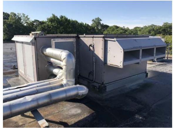
RIVE007e 5/13/2021 Makeup air handling unit Roof
