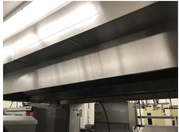
RIVE023e 5/13/2021 Commercial kitchen hood Room 158
