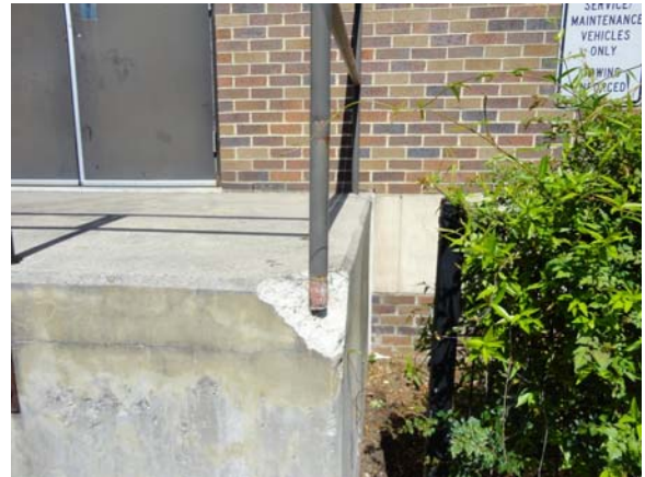
RIVE088a 5/13/2021 Damaged rail anchor at new service dock Southeast elevation
