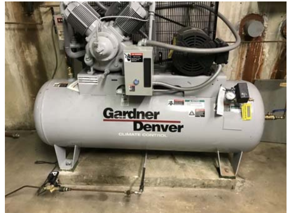
RIVE044e 5/13/2021 Controls air compressor Room 03
