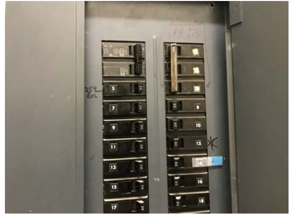
RIVE010e 5/13/2021 Local panelboard Second floor, electrical room
