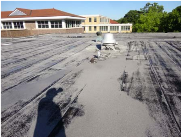
RIVE007a 5/13/2021 Heavy weathering of granular finish on cap sheet Main roof
