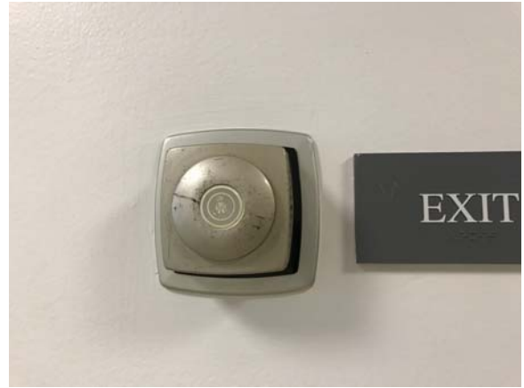
RIVE037e 5/13/2021 Pneumatic local thermostat First floor corridor
