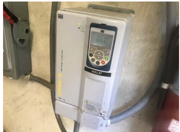
RIVE060e 5/13/2021 VFD for AHU-007 Room 05
