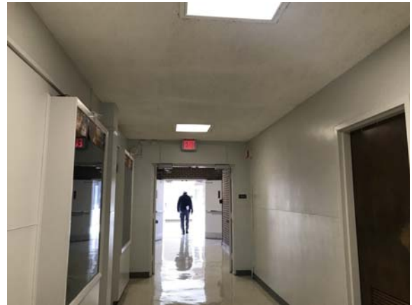
RIVE011e 5/13/2021 Retrofitted LED lighting fixtures Second floor corridor
