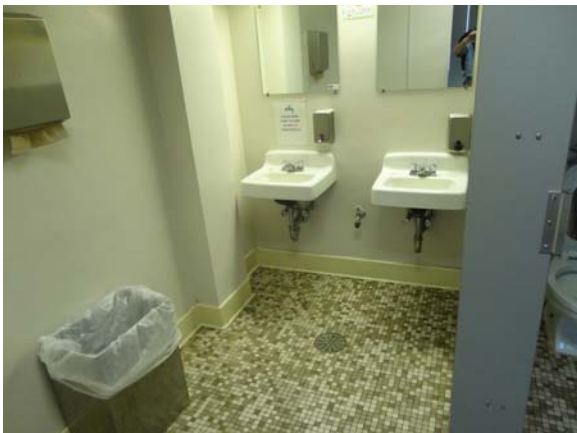
RIVE036a 5/13/2021 Older wall-hung lavatories Second floor, central women's restroom
