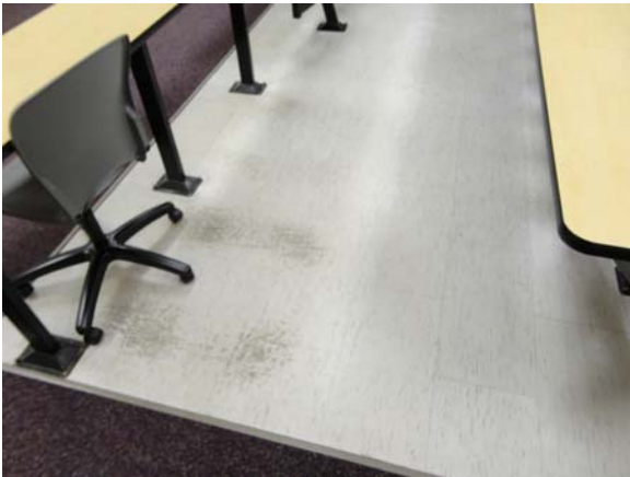
RIVE065a 5/13/2021 Worn vinyl flooring in seating aisles First floor, north lecture room
