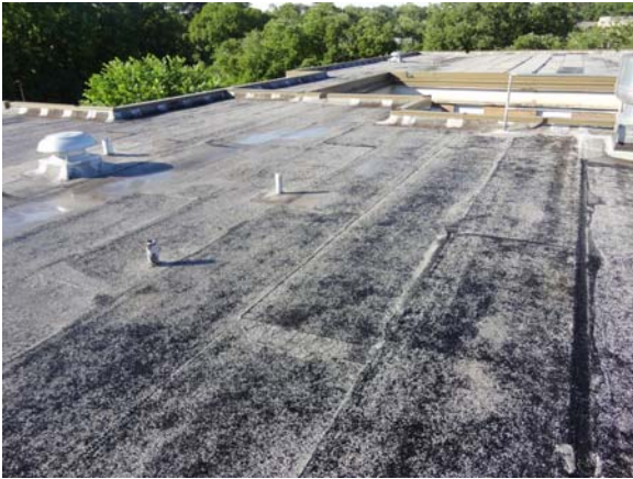
RIVE001a 5/13/2021 Weathered built-up roof with cap sheet Main roof
