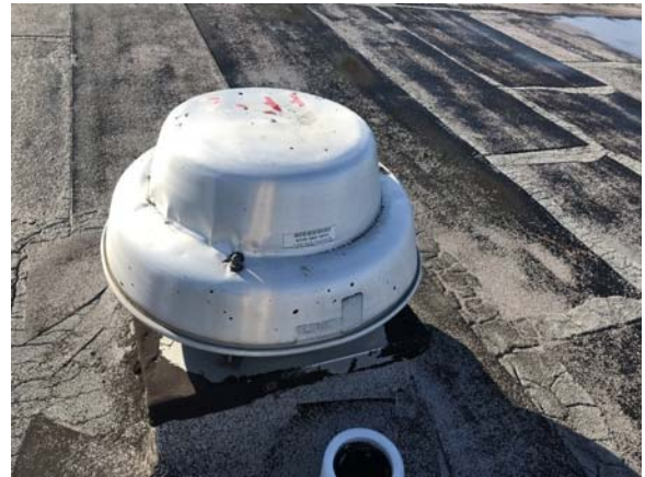
RIVE002e 5/13/2021 Centrifugal rooftop exhaust fan Roof
