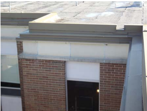
RIVE003a 5/13/2021 Staining and weathered caulking Upper precast concrete banding
