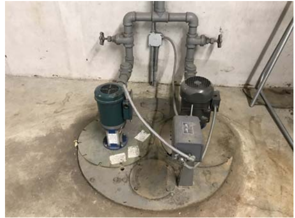
RIVE058e 5/13/2021 Sump pump Room 04
