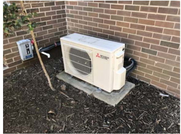
RIVE052e 5/13/2021 Ductless split condensing unit Site
