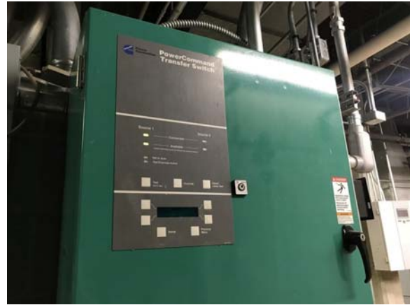
RIVE049e 5/13/2021 Automatic transfer switch Room 03
