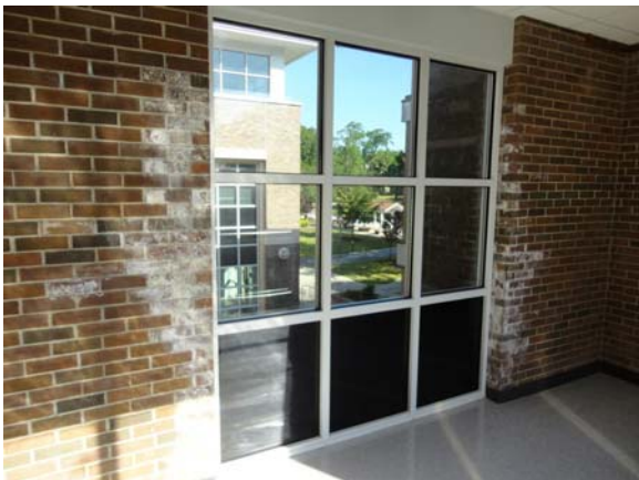
RIVE039a 5/13/2021 Some efflorescence around exterior glazing Second floor, north corridor
