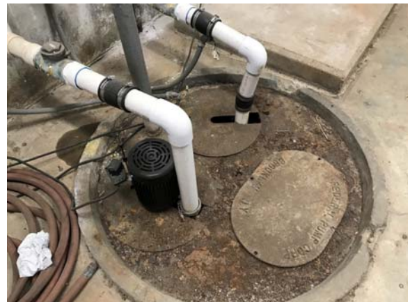
RIVE042e 5/13/2021 Sump pump Room 03
