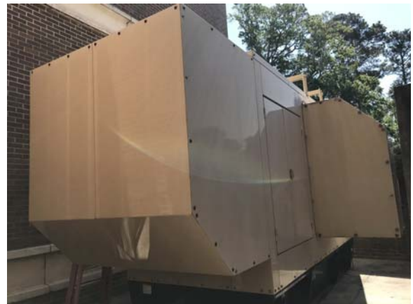
RIVE054e 5/13/2021 Emergency generator Site
