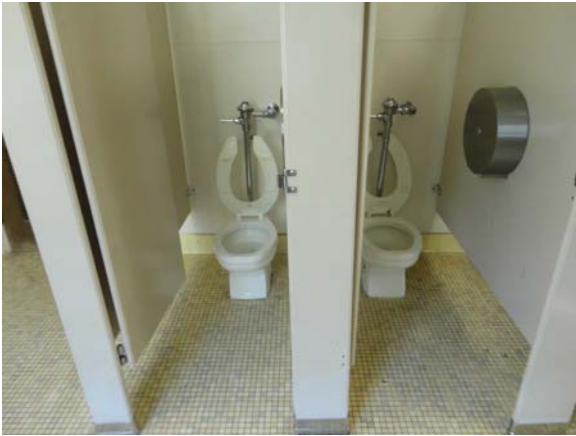
RIVE016a 5/13/2021 Older standard tankless water closets Second floor, south women's restroom
