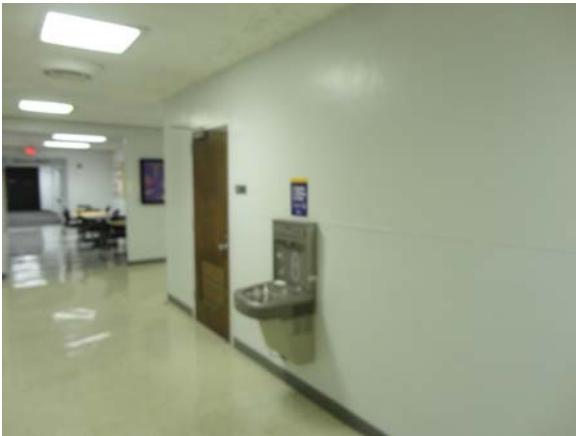
RIVE029a 5/13/2021 Newer single-level water fountain with bottle filler Second floor corridor
