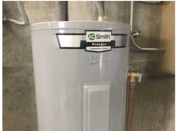
RIVE062e 5/13/2021 Residential electric water heater Room 05
