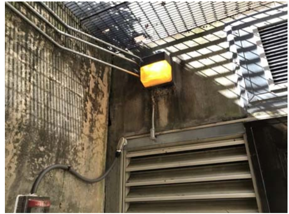
RIVE041e 5/13/2021 HID wallpack Areaway
