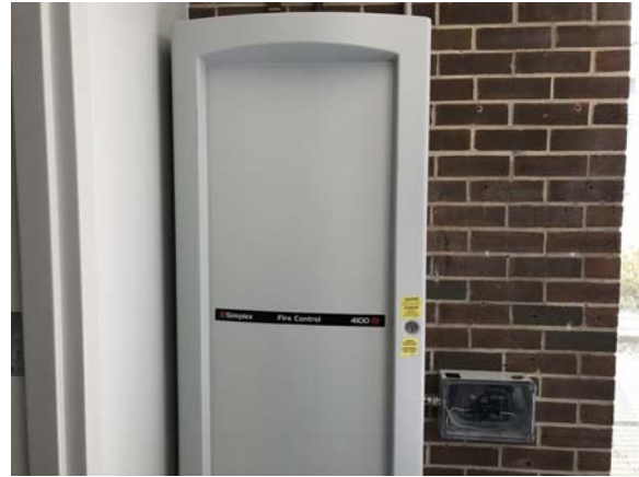
RIVE028e 5/13/2021 Fire alarm extension panel First floor corridor
