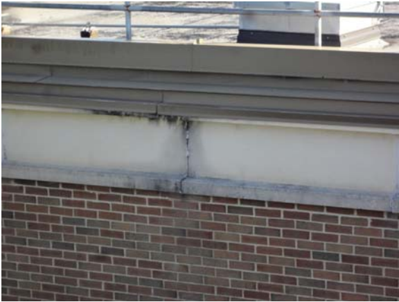
RIVE004a 5/13/2021 Stained and weathered caulking Upper precast concrete banding
