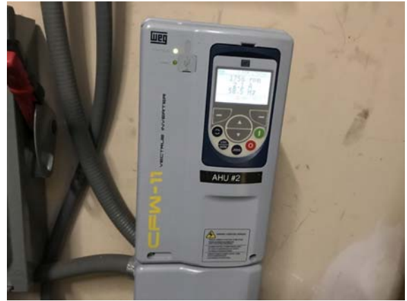
RIVE031e 5/13/2021 VFD for AHU-002 Room 113
