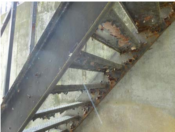
RIVE089a 5/13/2021 Peeling paint on areaway steps Typical areaway
