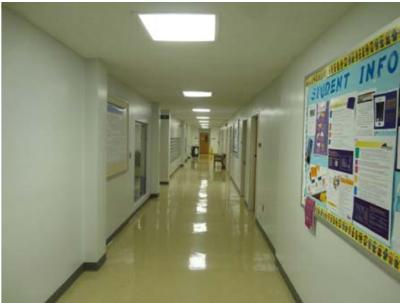
RIVE059a 5/13/2021 Older vinyl floor tile and original textured ceiling First floor corridor
