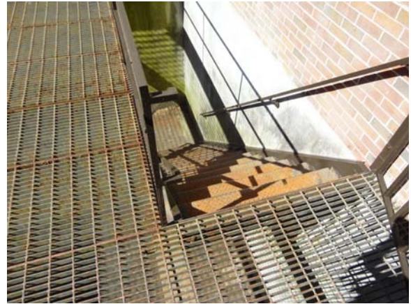
RIVE074a 5/13/2021 Rusted areaway access steps Courtyard
