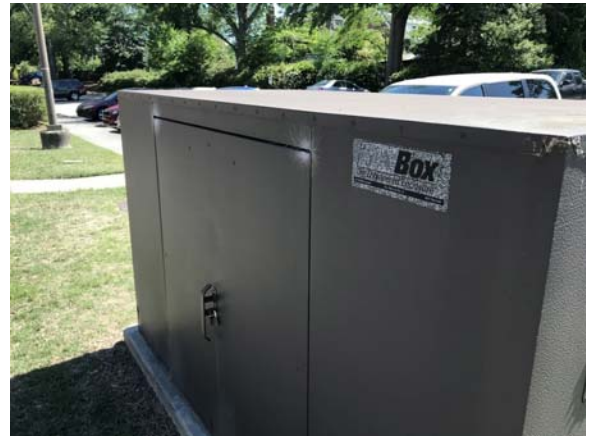
RIVE059e 5/13/2021 Location of water main backflow preventers Site
