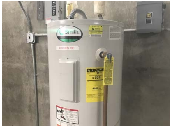
RIVE063e 5/13/2021 Residential electric water heater Room 05
