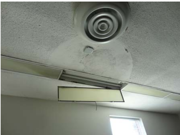
RIVE027a 5/13/2021 Damaged textured ceiling Second floor, textile lab
