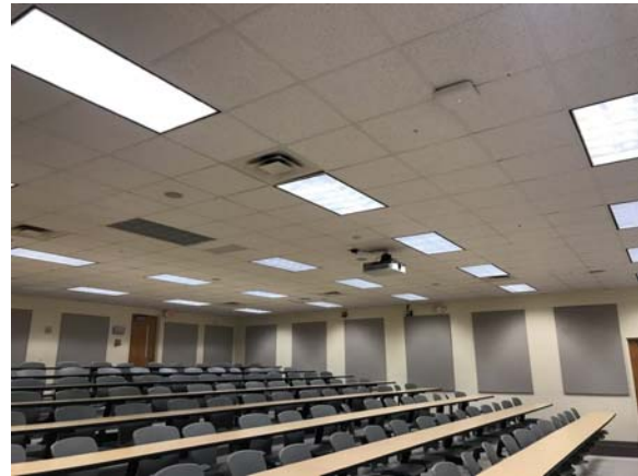
RIVE029e 5/13/2021 Open-cell grid T8 lighting fixtures Room 102
