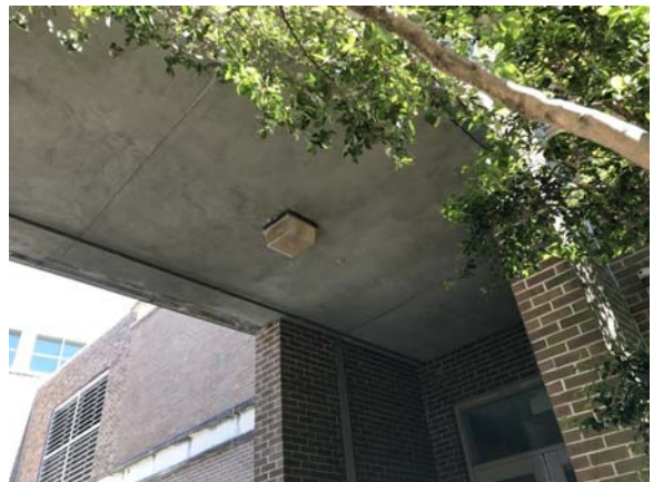
RIVE066e 5/13/2021 Ceiling-mounted HID lighting fixture Exterior soffit
