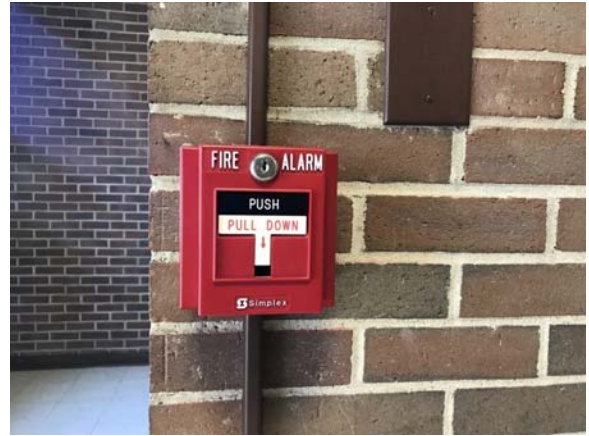
RIVE013e 5/13/2021 Manual pull fire alarm device Second floor corridor
