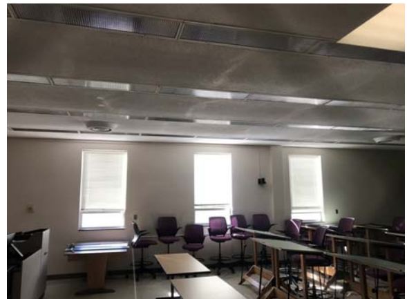
RIVE012e 5/13/2021 Original retrofitted T8 lighting fixtures Room 262
