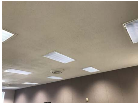
RIVE020e 5/13/2021 Original retrofitted T8 lighting fixtures Room 253
