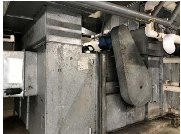
RIVE056e 5/13/2021 Air handling unit AHU-006 Room 04
