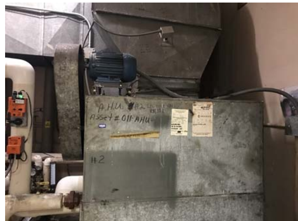
RIVE030e 5/13/2021 Air handling unit AHU-002 Room 113
