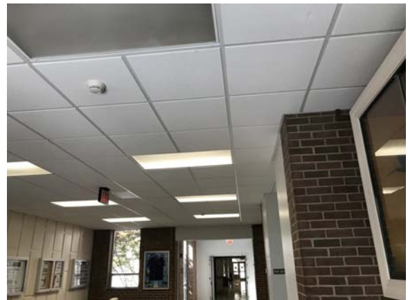
RIVE027e 5/13/2021 Recessed T8 lighting fixtures First floor corridor
