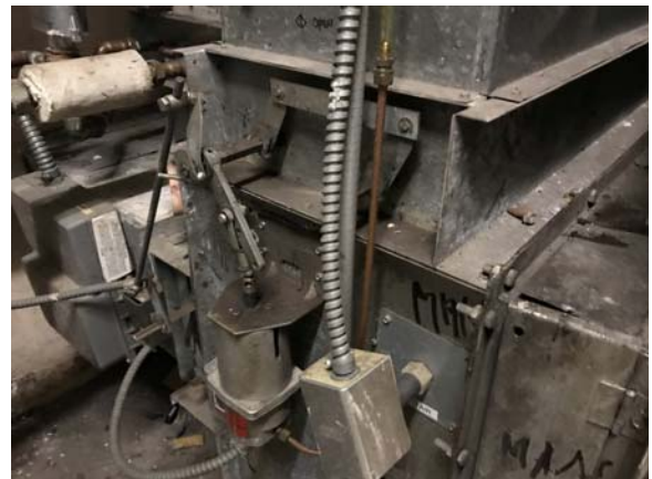
RIVE033e 5/13/2021 Air handling unit AHU-003 Room 113
