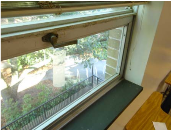
RIVE020a 5/13/2021 Original single-pane, metal-framed glazing Second floor
