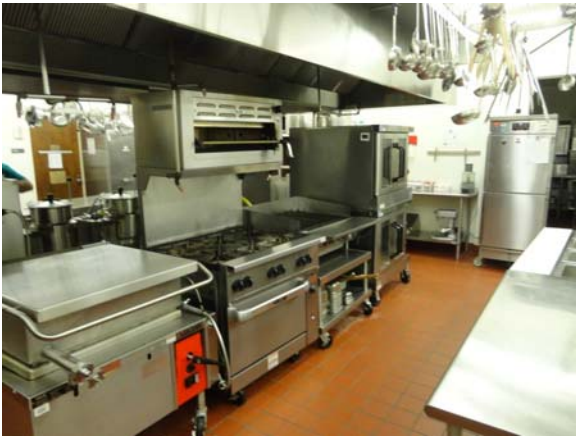
RIVE056a 5/13/2021 Cooking equipment First floor, east Culinary area
