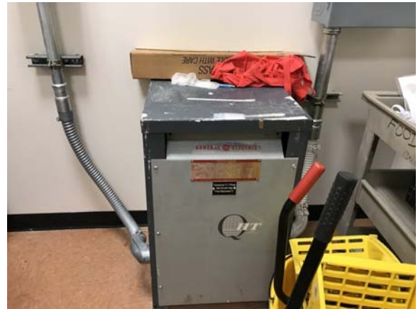
RIVE026e 5/13/2021 Secondary step-down transformer Room 158
