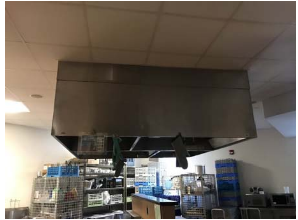
RIVE025e 5/13/2021 Commercial kitchen hood Room 158
