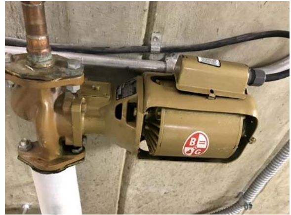
RIVE046e 5/13/2021 Domestic hot water circulation pump Room 03
