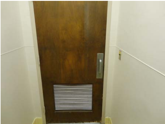
RIVE017a 5/13/2021 Narrow clearances in restroom vestibules Second floor, restrooms
