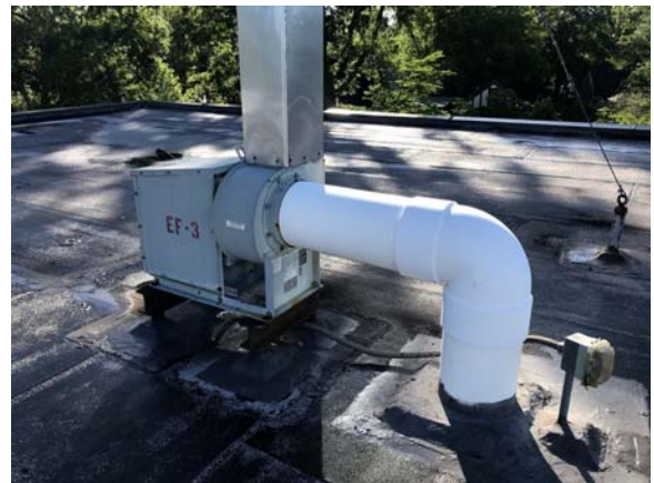
RIVE003e 5/13/2021 Utility-style exhaust fan Roof
