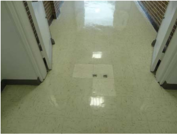
RIVE010a 5/13/2021 Older vinyl flooring with dissimilar tile repair Second floor corridor
