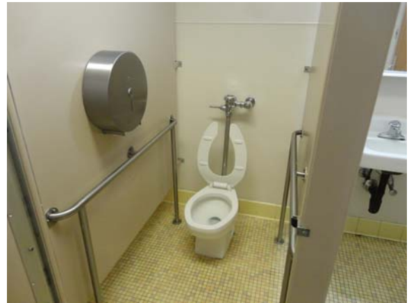
RIVE070a 5/13/2021 Partially accessible toilet stall First floor, men's restroom
