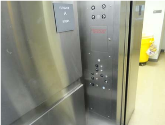
RIVE067a 5/13/2021 Accessible elevator control panel Passenger elevator cab
