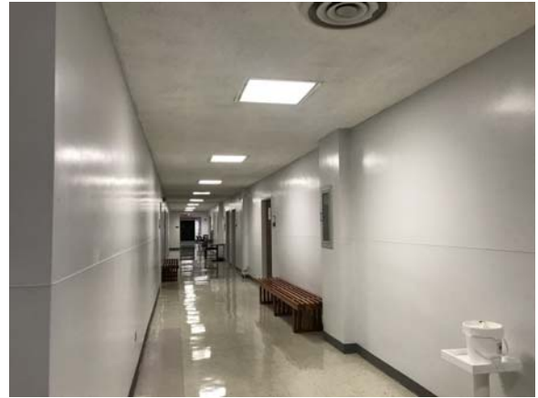
RIVE016e 5/13/2021 Retrofitted LED lighting fixtures Second floor corridor
