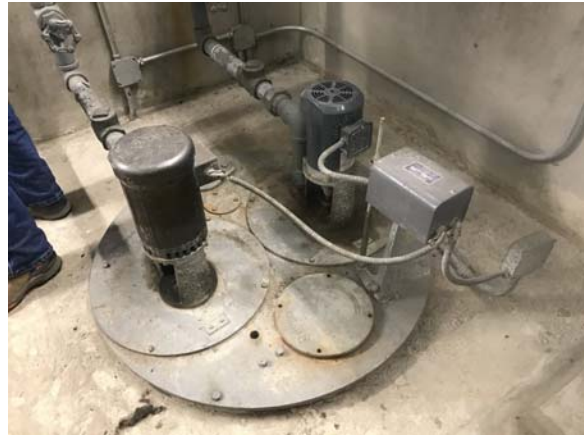
RIVE064e 5/13/2021 Sump pump Room 05
