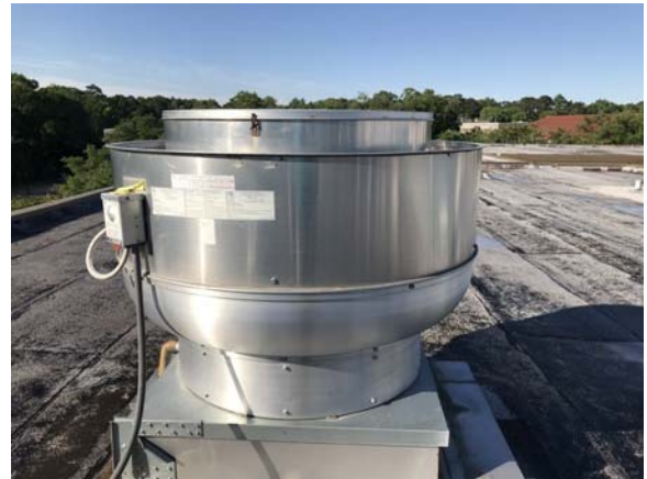
RIVE005e 5/13/2021 Kitchen exhaust fan Roof
