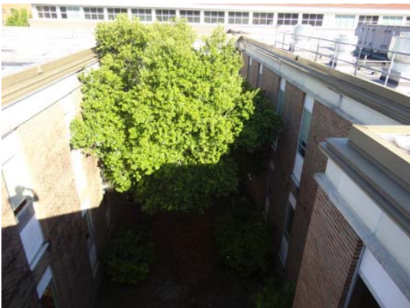
RIVE009a 5/13/2021 Tree in courtyard restricting access for facade cleaning Exterior courtyard
