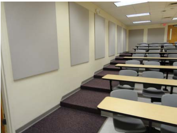
RIVE063a 5/13/2021 No side aisle handrails or assistive listening First floor, north lecture room
