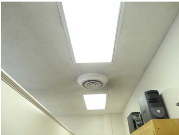
RIVE024a 5/13/2021 Original textured ceiling Second floor, south office suite
