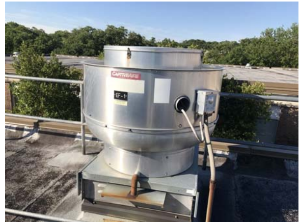
RIVE008e 5/13/2021 Kitchen exhaust fan Roof
