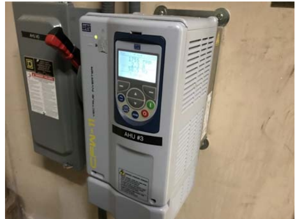
RIVE032e 5/13/2021 VFD for AHU-003 Room 113
