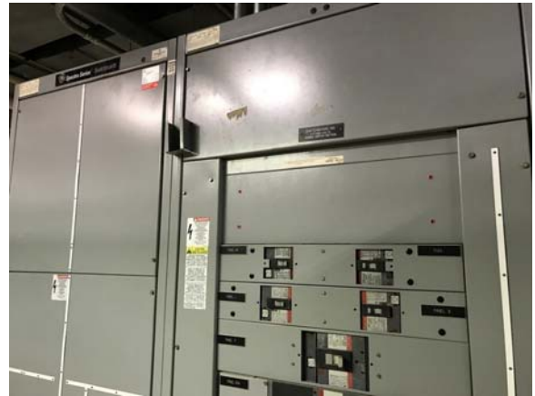
RIVE047e 5/13/2021 Main switchboard Room 03
