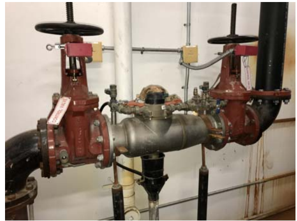
SCIT061e 5/10/2021 Backflow preventer for fire suppression Room C101
