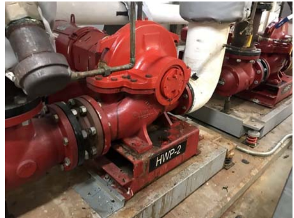
SCIT029e 5/10/2021 Heating hot water pumps Room P01
