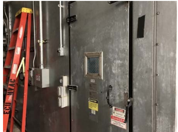
SCIT035e 5/10/2021 Air handling unit AHU-7 Room P05
