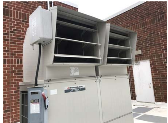
SCIT033e 5/10/2021 VRF condensing units Roof
