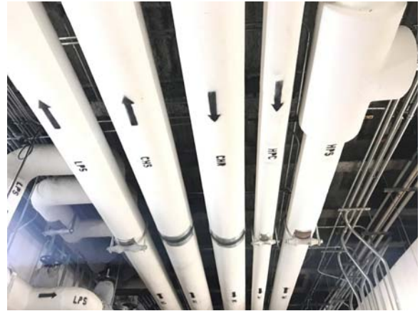
SCIT025e 5/10/2021 Insulated mechanical piping Room P01
