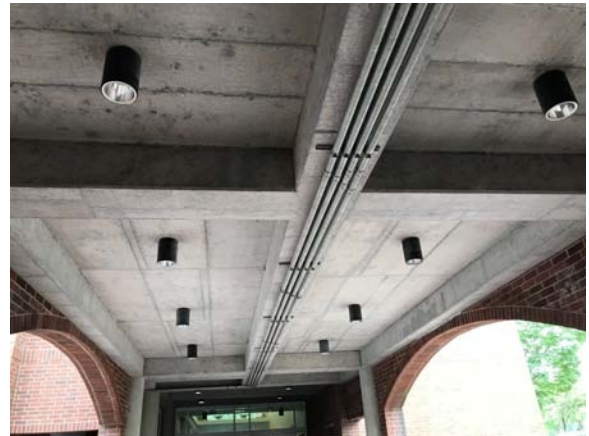
SCIT080e 5/10/2021 Ceiling-mounted lighting fixtures Exterior soffit
