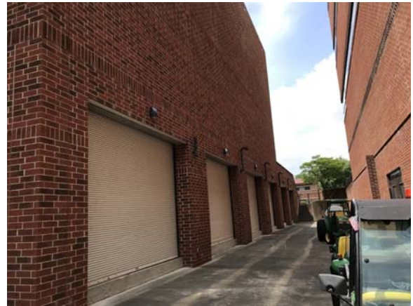
SCIT074e 5/10/2021 LED sconce lighting fixtures Exterior
