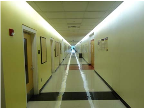
SCIT024a 5/10/2021 Vinyl floor tile, painted walls, and acoustical ceiling Fifth floor corridor
