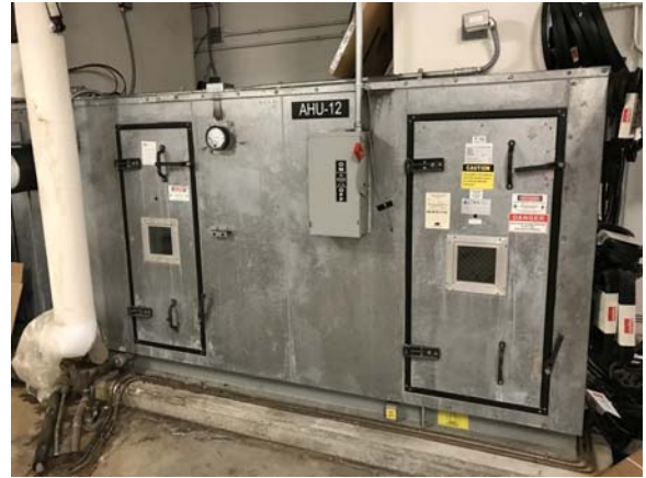
SCIT064e 5/10/2021 Air handling unit AHU-12 Room C101
