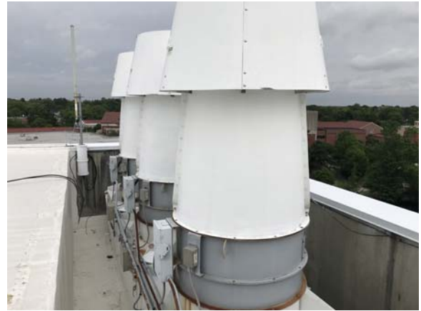
SCIT004e 5/10/2021 Short stack, mixed flow exhaust fans Roof
