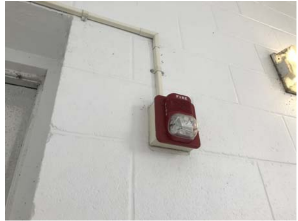
SCIT037e 5/10/2021 Horn with strobe fire alarm device Fifth floor corridor
