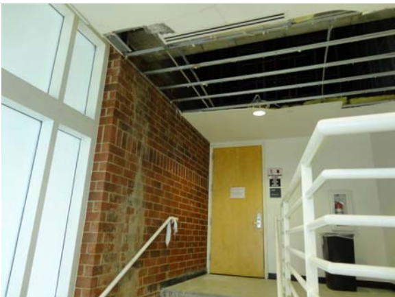
SCIT075a 5/10/2021 Unrepaired ceiling damage Third floor, north classroom wing commons
