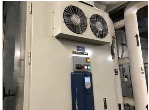
SCIT024e 5/10/2021 VFD for AHU-1 Room P01
