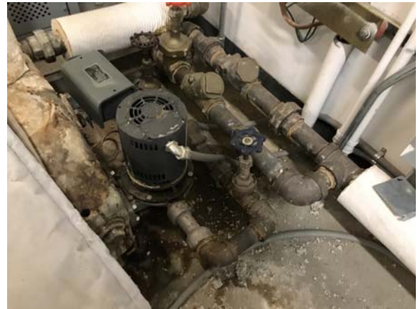
SCIT026e 5/10/2021 Condensate receiver Room P01
