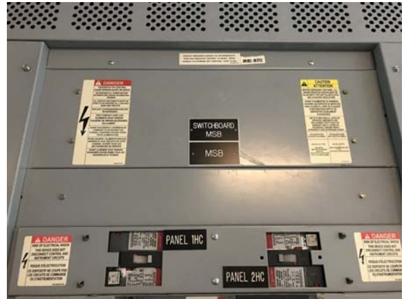
SCIT071e 5/10/2021 Main switchboard Room C102
