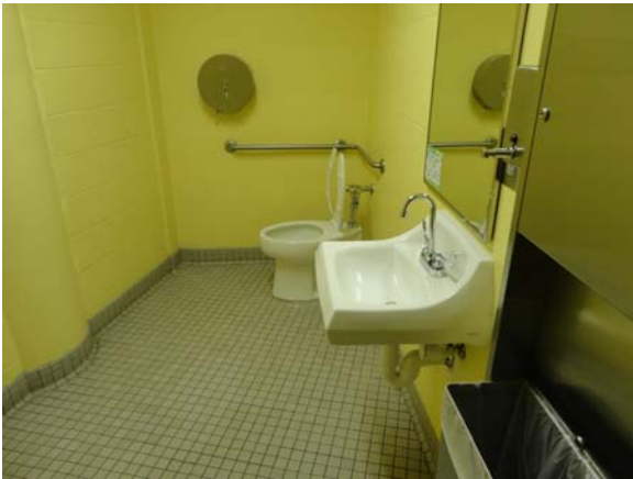
SCIT091a 5/10/2021 Accessible wall-hung lavatory and tankless water closet First floor, central plant bath
