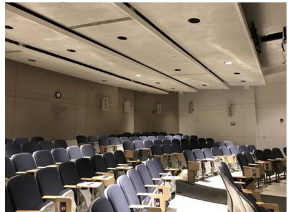
SCIT057e 5/10/2021 Recessed can CFL lighting fixtures Room C309
