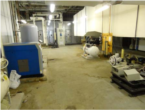
SCIT010a 5/10/2021 Concrete floor needs to be resealed Upper penthouse interior
