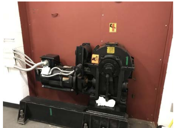
SCIT075e 5/10/2021 Elevator traction gear Room 128A
