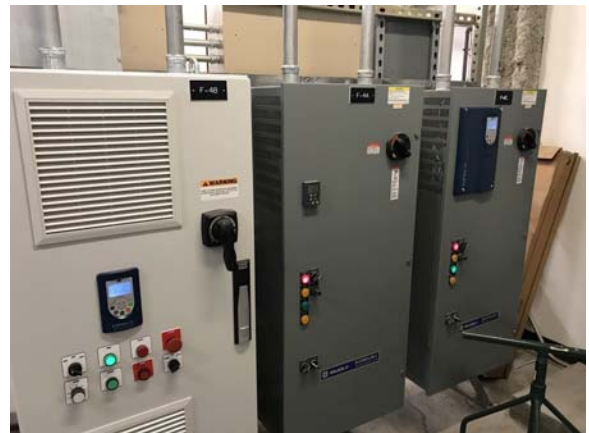
SCIT012e 5/10/2021 VFDs for short stack, mixed flow exhaust fans Room P01
