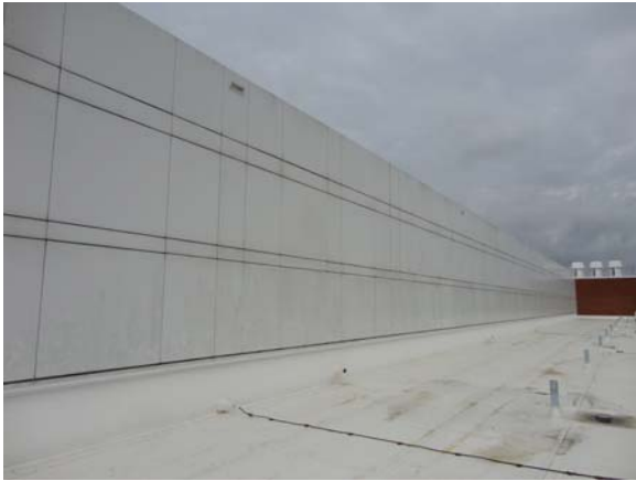
SCIT013a 5/10/2021 Some staining on prefinished metal siding Upper penthouse
