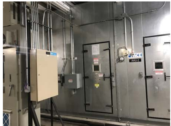
SCIT021e 5/10/2021 Air handling unit AHU-2 Room P01
