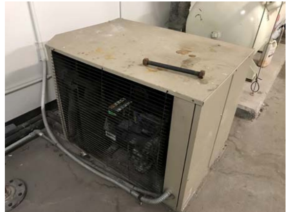
SCIT008e 5/10/2021 Condenser for walk-in cooler Room P01
