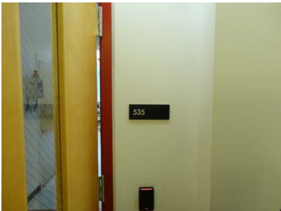
SCIT027a 5/10/2021 Smart card locks for lab entry doors Fifth floor corridor
