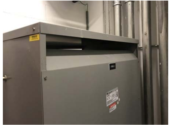
SCIT040e 5/10/2021 Secondary step-down transformer Room 529
