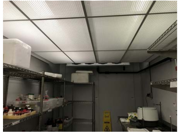
SCIT046e 5/10/2021 Interior of walk-in cooler Cold room 446
