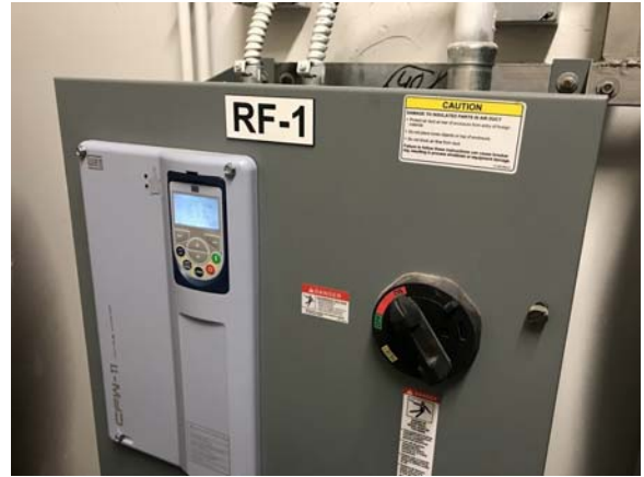
SCIT034e 5/10/2021 VFD for RF-1 Room P05
