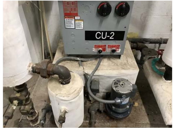
SCIT067e 5/10/2021 Condensate receiver Room C101
