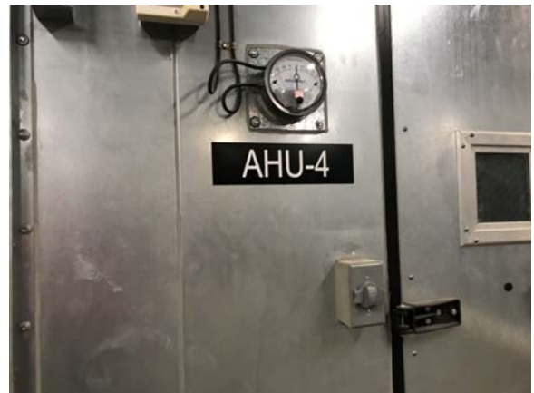
SCIT018e 5/10/2021 Air handling unit AHU-4 Room P01
