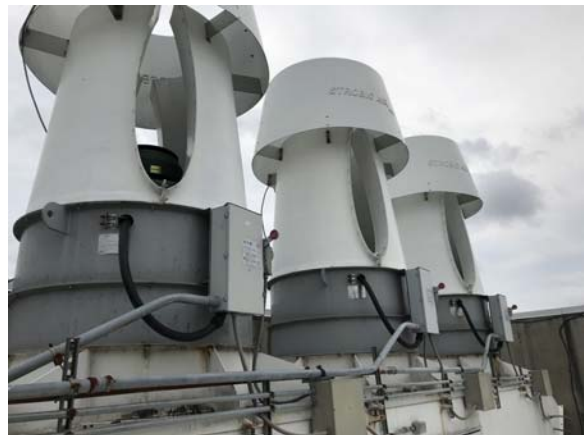
SCIT003e 5/10/2021 Short stack, mixed flow exhaust fans Roof
