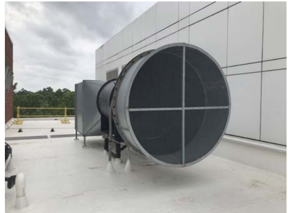
SCIT032e 5/10/2021 Smoke exhaust fan Roof
