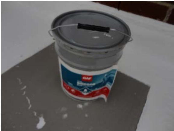
SCIT065a 5/10/2021 Membrane getting coated to prolong its life span Breezeway link to classroom building
