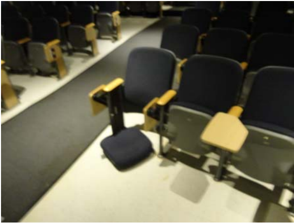
SCIT079a 5/10/2021 Seat damage in lecture hall Third floor, north lecture hall
