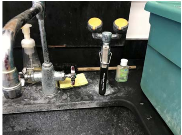
SCIT044e 5/10/2021 Typical sink-mounted emergency eyewash station Room 531
