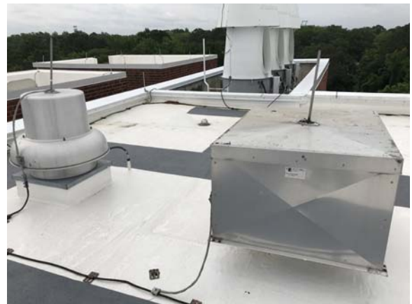
SCIT006e 5/10/2021 Centrifugal rooftop exhaust fan Roof
