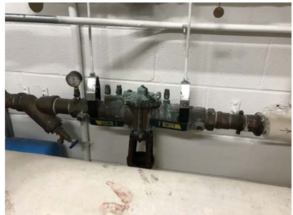
SCIT030e 5/10/2021 Backflow preventer Room P01
