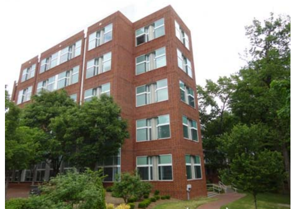
SCIT100a 5/10/2021 Exterior brick facade and glazing Southwest corner elevation of south wing
