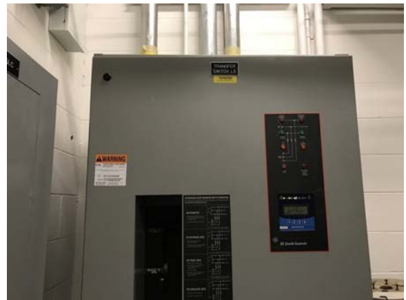
SCIT072e 5/10/2021 Automatic transfer switch Room C102
