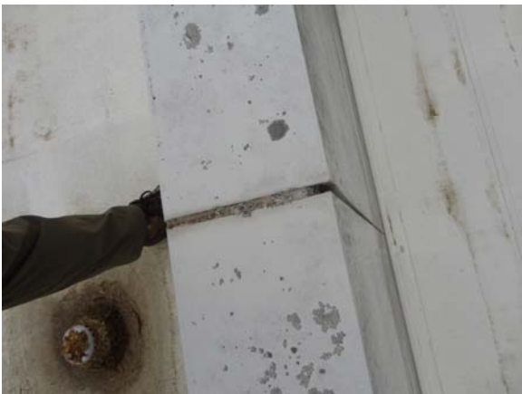
SCIT006a 5/10/2021 Weathered caulk joint Upper roof parapet
