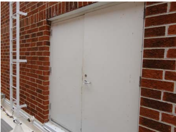
SCIT009a 5/10/2021 Hollow-metal service doors Upper penthouse
