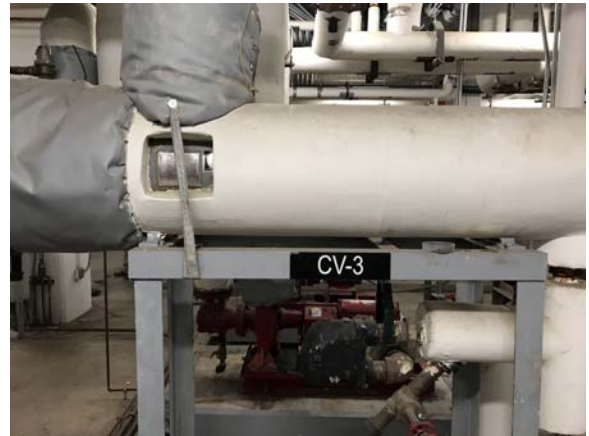
SCIT068e 5/10/2021 Heating hot water shell-and-tube heat exchanger Room C101
