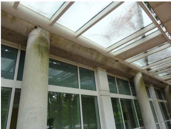
SCIT105a 5/10/2021 Staining on lower exterior facade South elevation of south wing
