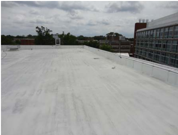
SCIT068a 5/10/2021 Weathered membrane roof on classroom building North classroom membrane roof
