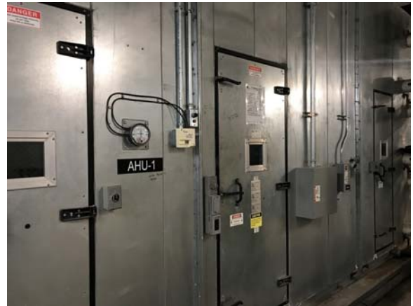
SCIT023e 5/10/2021 Air handling unit AHU-1 Room P01
