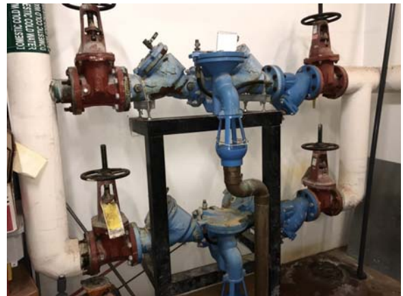
SCIT060e 5/10/2021 Backflow preventers Room C101
