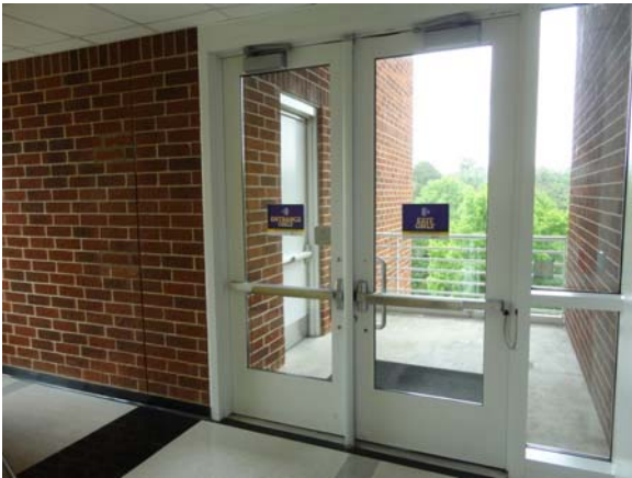
SCIT035a 5/10/2021 Glass egress doors to exterior stair tower Fifth floor, southeast stair tower
