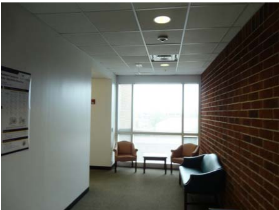
SCIT030a 5/10/2021 Original broadloom carpeting and acoustical ceiling Fifth floor, west office area
