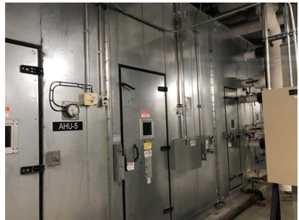
SCIT015e 5/10/2021 Air handling unit AHU-5 Room P01
