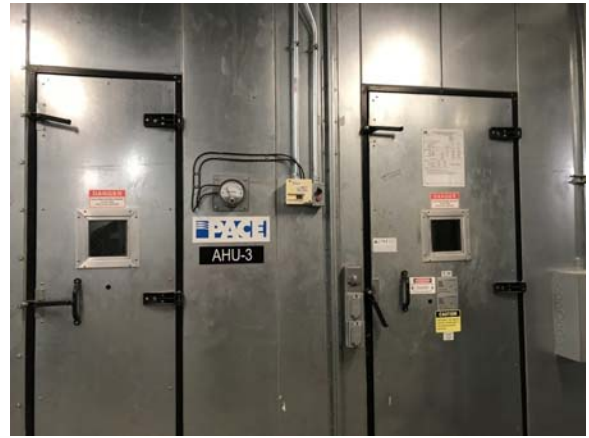
SCIT020e 5/10/2021 Air handling unit AHU-3 Room P01
