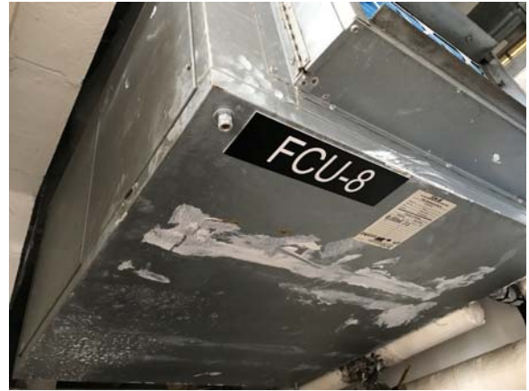
SCIT055e 5/10/2021 Typical fan coil unit Room C305
