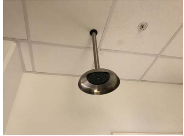
SCIT041e 5/10/2021 Typical emergency shower Room 530
