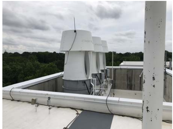
SCIT002e 5/10/2021 Short stack, mixed flow exhaust fans Roof
