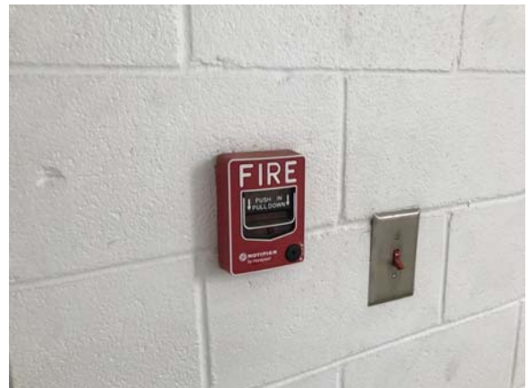
SCIT036e 5/10/2021 Manual pull fire alarm device Fifth floor corridor
