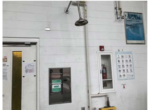
SCIT053e 5/10/2021 Combination emergency shower and eyewash station Room 144A
