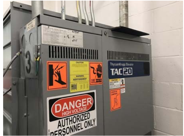
SCIT079e 5/10/2021 Hydraulic elevator controls Room 156
