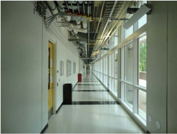
SCIT052a 5/10/2021 Vinyl flooring and no formal ceiling in corridor First floor, south perimeter corridor
