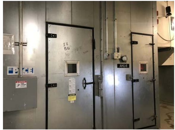
SCIT014e 5/10/2021 Air handling unit AHU-6 Room P01
