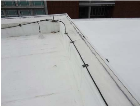
SCIT067a 5/10/2021 Failing parapet membrane Breezeway link to classroom building
