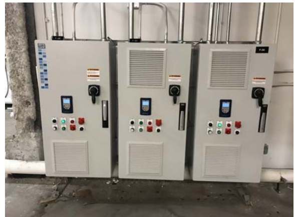
SCIT027e 5/10/2021 VFDs for short stack, mixed flow exhaust fans Room P01
