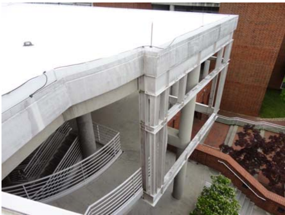
SCIT069a 5/10/2021 Staining on ornamental steel work North breezeway
