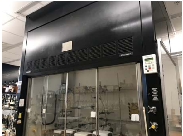
SCIT043e 5/10/2021 Typical laboratory fume hood Room 531
