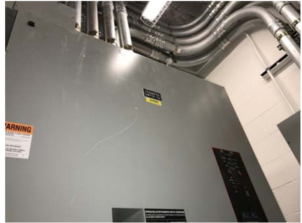
SCIT073e 5/10/2021 Automatic transfer switch Room C102
