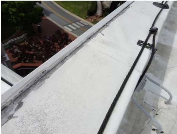
SCIT064a 5/10/2021 Heavily weathered membrane roof Breezeway link to classroom building
