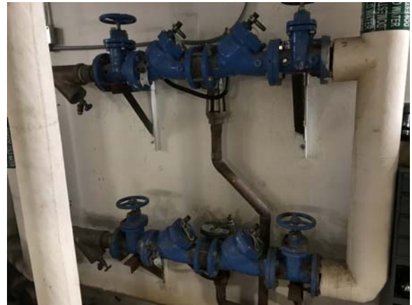
SCIT059e 5/10/2021 Backflow preventers Room C101
