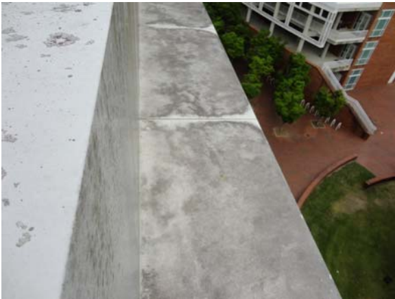
SCIT011a 5/10/2021 Signs of water ponding on outer metal solar screen Upper exterior facade
