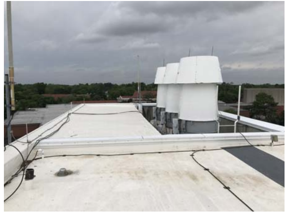
SCIT001e 5/10/2021 Short stack, mixed flow exhaust fans Roof
