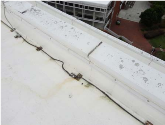
SCIT004a 5/10/2021 Weathered caulking on metal cap Penthouse roof
