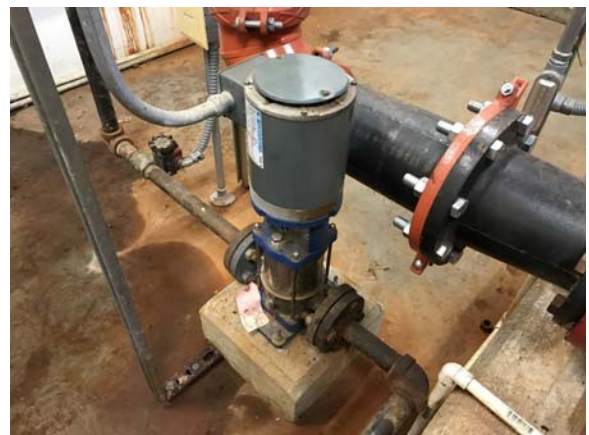
SCIT063e 5/10/2021 Jockey pump Room C101
