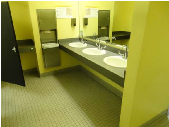
SCIT018a 5/10/2021 Counter lavatories Fifth floor, west women's restroom
