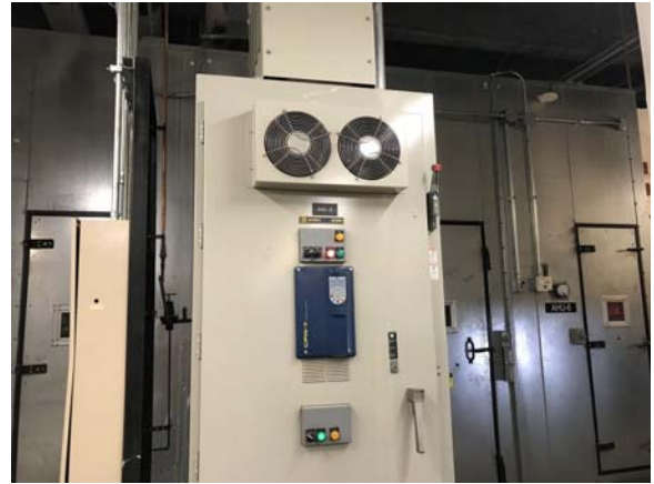
SCIT013e 5/10/2021 VFD for AHU-6 Room P01
