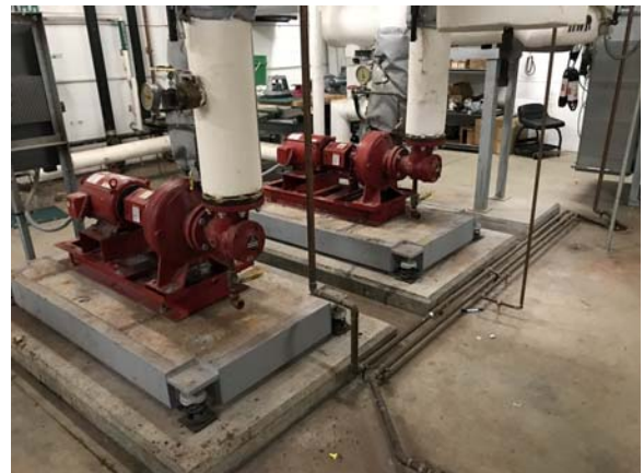
SCIT066e 5/10/2021 Heating hot water pumps Room C101
