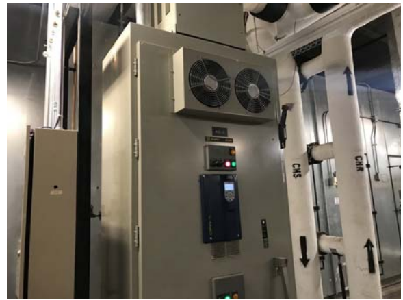
SCIT019e 5/10/2021 VFD for AHU-3 Room P01
