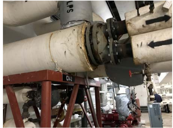
SCIT028e 5/10/2021 Heating hot water shell-and-tube heat exchanger Room P01
