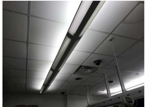
SCIT038e 5/10/2021 Suspended T8 lighting fixtures Room 519
