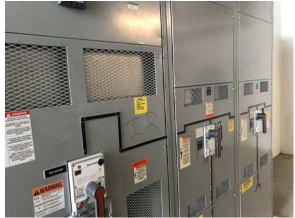
SCIT070e 5/10/2021 Load interrupter Room C102
