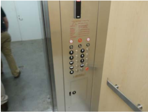
SCIT001a 5/10/2021 Accessible elevator control panel Passenger elevator cab
