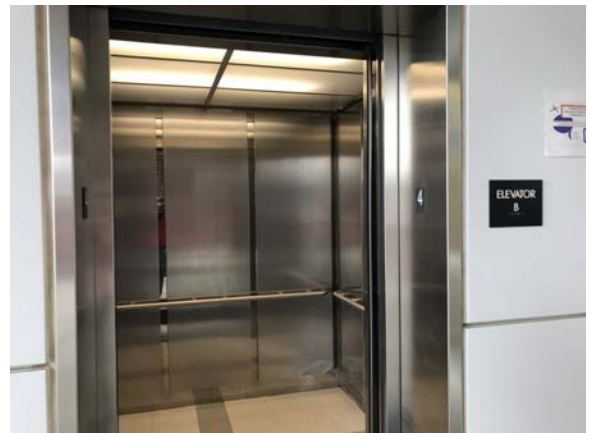
SCIT048e 5/10/2021 Elevator A interior Elevator A
