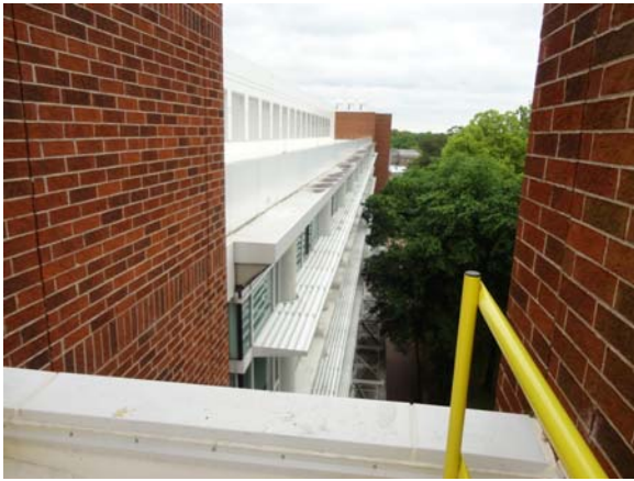
SCIT014a 5/10/2021 Signs of water ponding on outer metal solar screen Upper exterior facade
