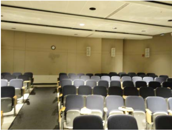
SCIT083a 5/10/2021 Cosmetic staining of rear acoustical wall panels Third floor, north lecture hall
