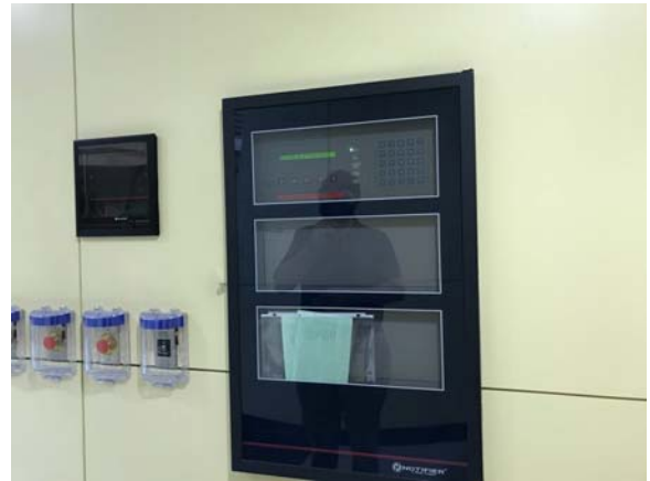
SCIT050e 5/10/2021 Main fire alarm panel First floor, lobby
