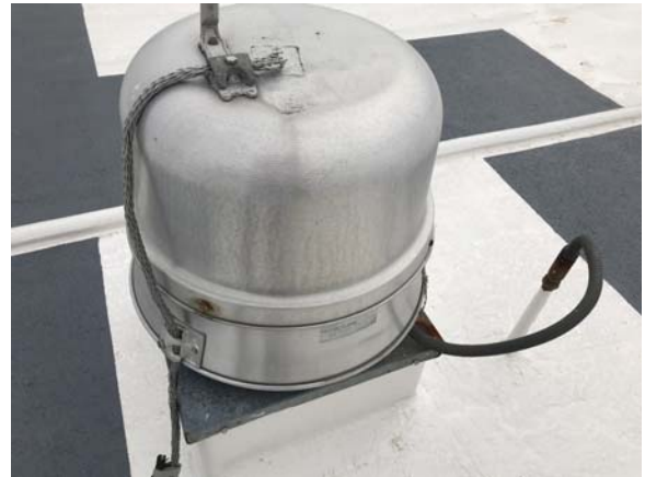
SCIT005e 5/10/2021 Centrifugal rooftop exhaust fan Roof
