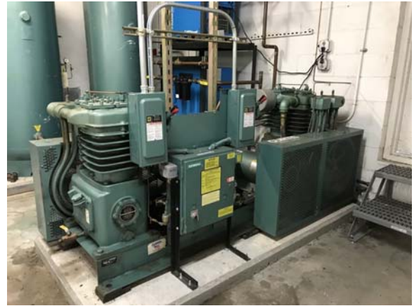
SCIT007e 5/10/2021 Laboratory air compressor Roof
