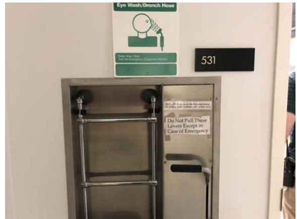
SCIT042e 5/10/2021 Typical emergency eyewash Room 530
