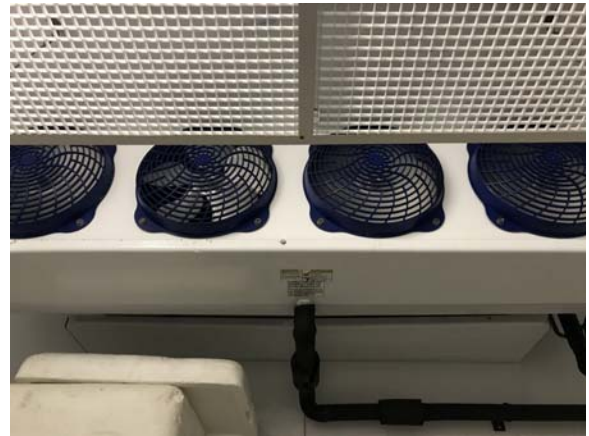
SCIT047e 5/10/2021 Typical walk-in cooler fan coil Cold room 446
