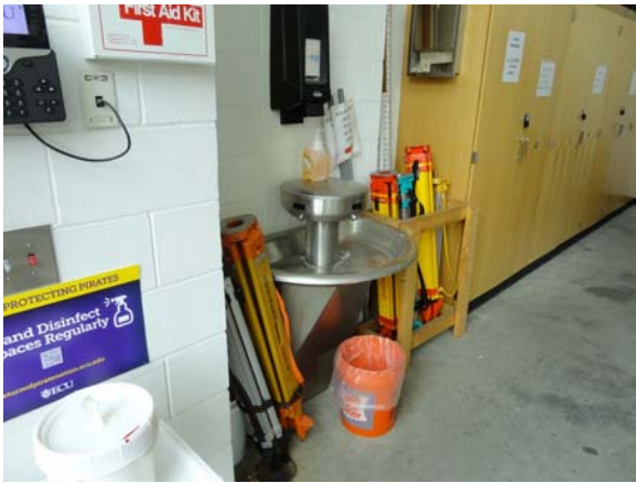
SCIT061a 5/10/2021 Stainless-steel trough sink First floor, ITEC high bay
