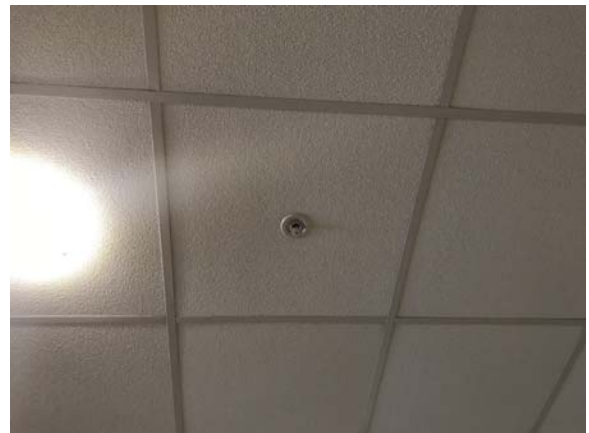
SCIT039e 5/10/2021 Fire suppression sprinkling device Room 519
