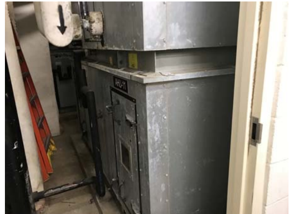
SCIT056e 5/10/2021 Air handling units AHU-10 and AHU-11 Room C308
