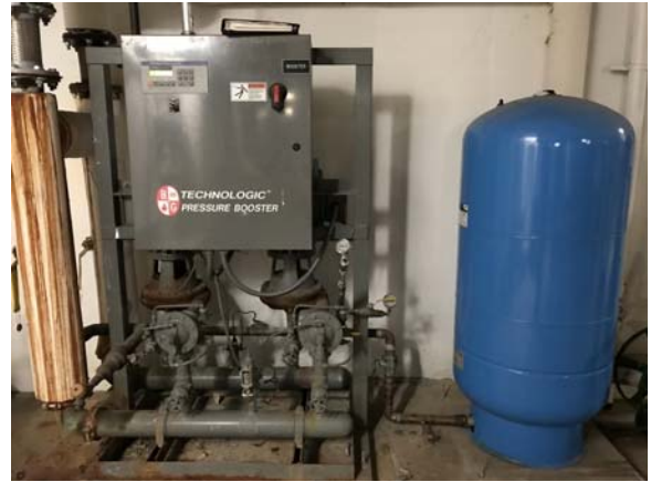
SCIT058e 5/10/2021 Domestic cold water booster pump system Room C101
