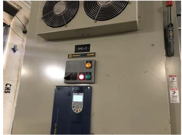
SCIT022e 5/10/2021 VFD for AHU-2 Room P01
