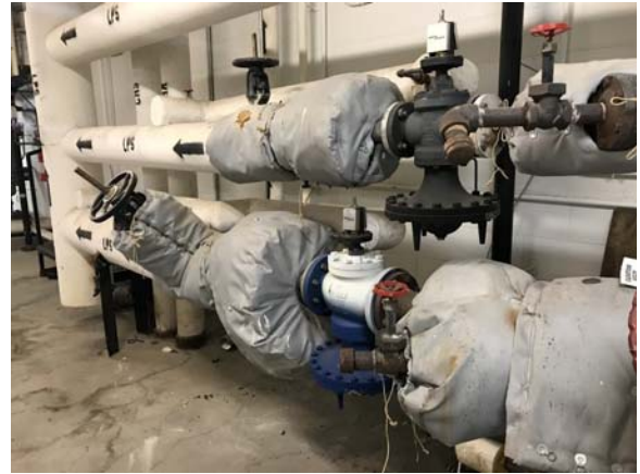
SCIT031e 5/10/2021 Pressure reducing valves Room P01
