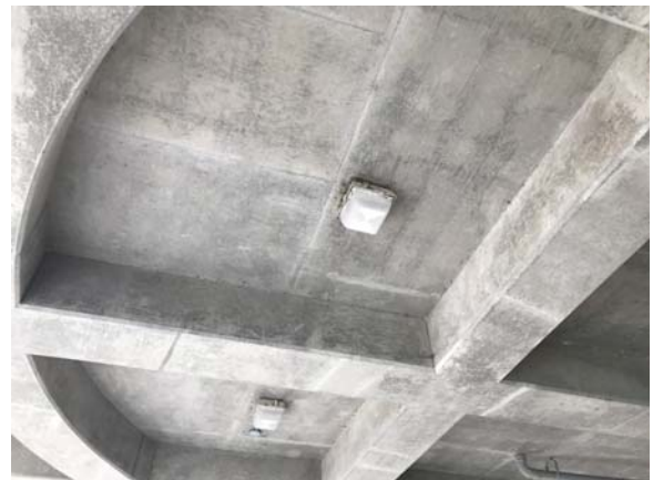
SCIT054e 5/10/2021 Ceiling-mounted HID lighting fixture Exterior soffit
