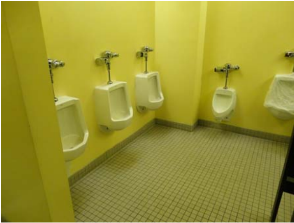
SCIT022a 5/10/2021 Wall-hung urinals Fifth floor, west men's restroom
