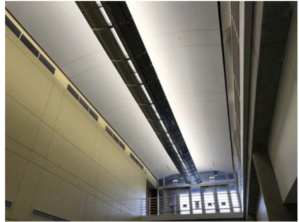
SCIT049e 5/10/2021 Upward diffusing T8 lighting fixtures Third floor corridor
