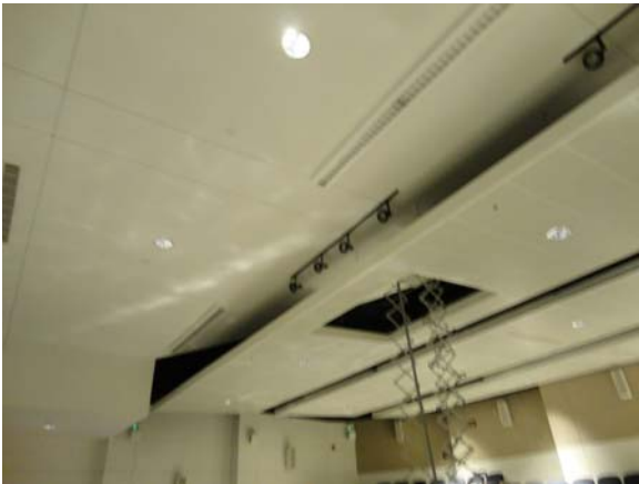
SCIT080a 5/10/2021 Painted ceiling Third floor, north lecture hall
