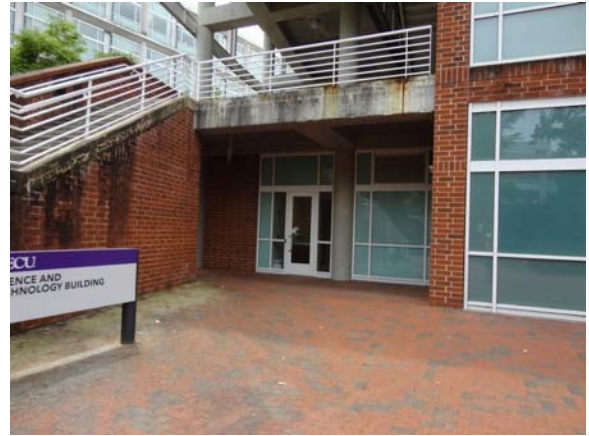
SCIT096a 5/10/2021 Localized heavy masonry staining East elevation of north wing
