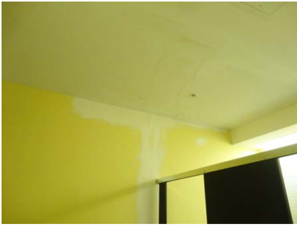
SCIT020a 5/10/2021 Unrepaired ceiling damage Fifth floor, west women's restroom
