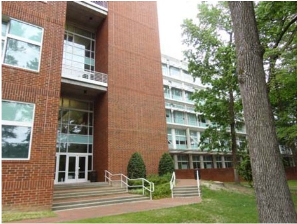
SCIT101a 5/10/2021 Exterior brick facade and glazing Southwest corner elevation of south wing
