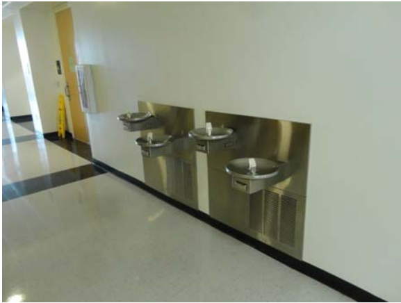
SCIT016a 5/10/2021 Two sets of dual-level water fountains Fifth floor, commons
