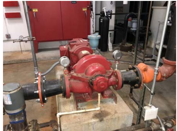
SCIT062e 5/10/2021 Main fire pump Room C101
