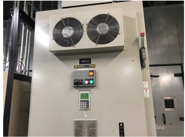
SCIT016e 5/10/2021 VFD for AHU-5 Room P01
