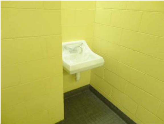
SCIT070a 5/10/2021 Accessible wall-hung lavatory North classroom wing men's restroom
