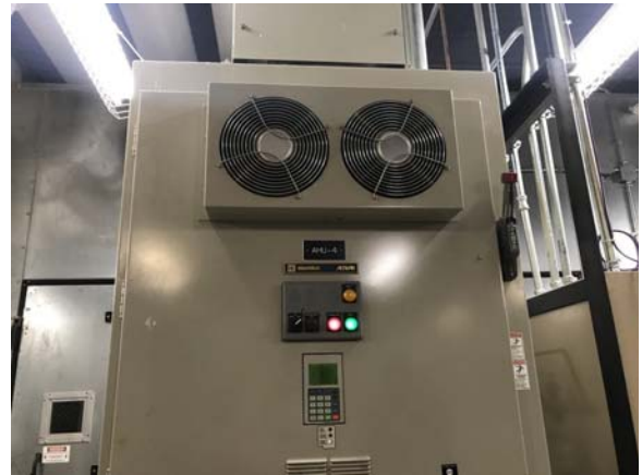
SCIT017e 5/10/2021 VFD for AHU-4 Room P01
