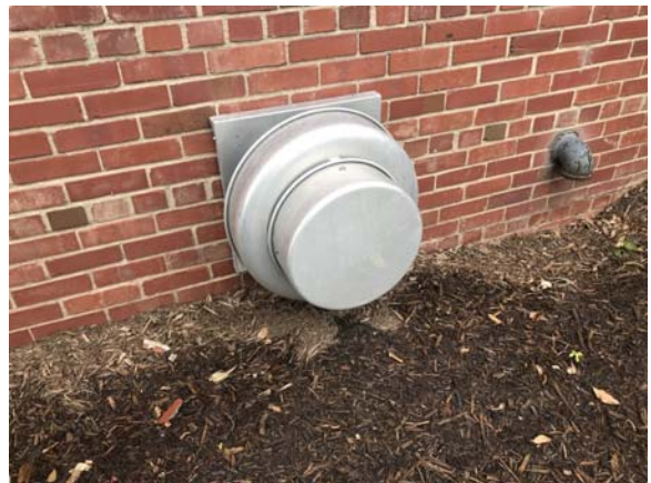
SLAY027e 5/12/2021 Centrifugal exhaust fan Exterior
