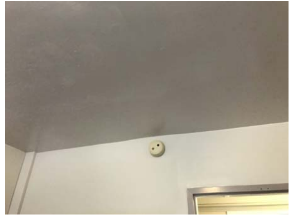
SLAY007e 5/12/2021 Smoke detector Room 348
