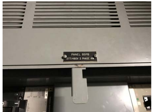
SLAY024e 5/12/2021 Main distribution panelboard Room 114E
