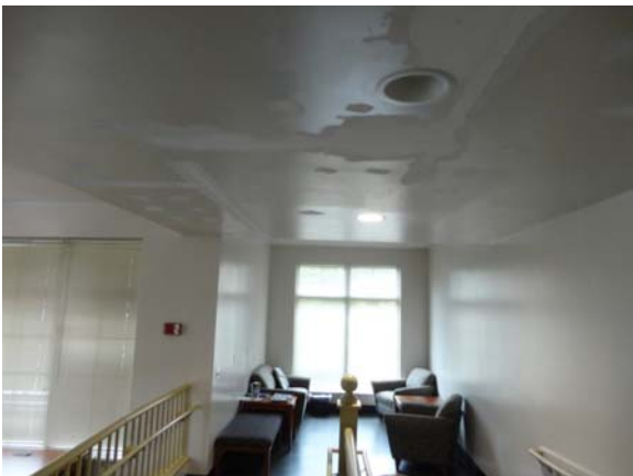
SLAY030a 5/12/2021 Unrepaired water damage to lobby ceiling First floor, entry lobby
