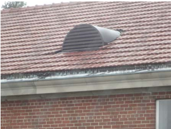
SLAY024a 5/12/2021 Pitched roof dormer vent and integral gutter Pitched clay tile main roof
