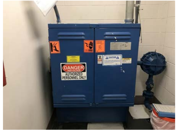
SLAY013e 5/12/2021 Hydraulic elevator controls Room 150
