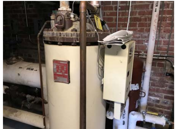
SLAY029e 5/12/2021 Domestic hot water heater exchanger Room 114E
