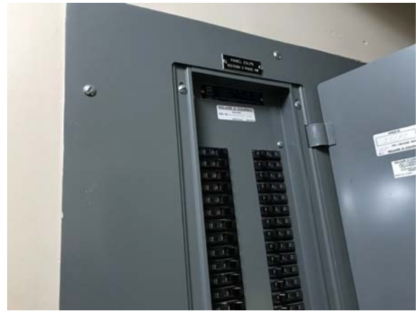
SLAY010e 5/12/2021 Local panelboard Second floor corridor
