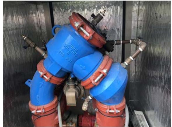
SLAY034e 5/12/2021 Fire suppression backflow preventer Exterior
