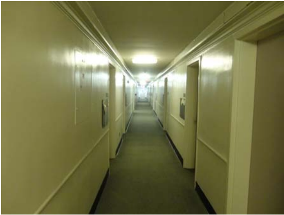
SLAY028a 5/12/2021 Worn carpeting and painted walls and ceiling First floor corridor
