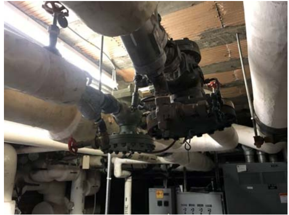
SLAY025e 5/12/2021 Pressure reducing valves Room 114E
