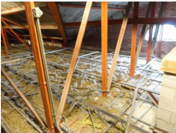
SLAY003a 5/12/2021 Inadequate insulation in attic Attic
