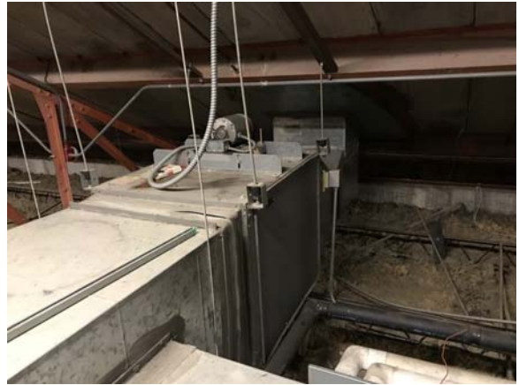
SLAY004e 5/12/2021 Inline centrifugal exhaust fan Attic
