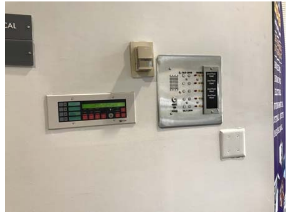
SLAY014e 5/12/2021 Fire alarm annunciator panel Main lobby
