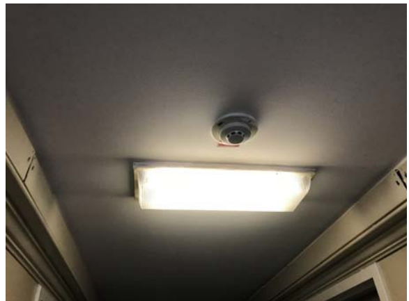
SLAY006e 5/12/2021 T8 troffer lighting fixture Third floor corridor
