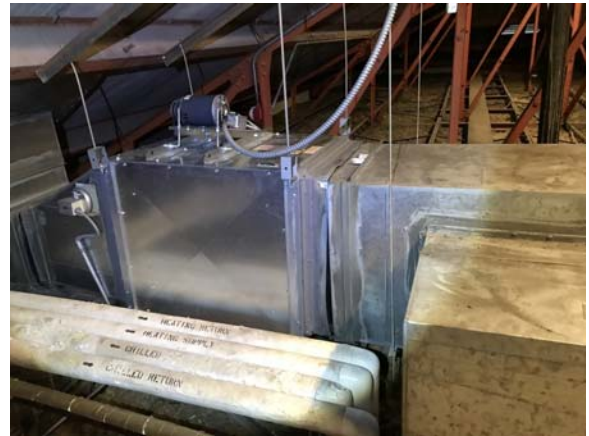
SLAY002e 5/12/2021 Inline centrifugal exhaust fan Attic
