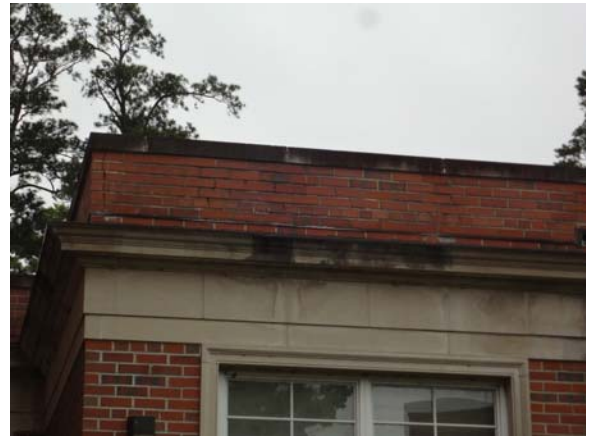
SLAY047a 5/12/2021 Stress cracks at corner of brick and staining of cut stone Upper east elevation
