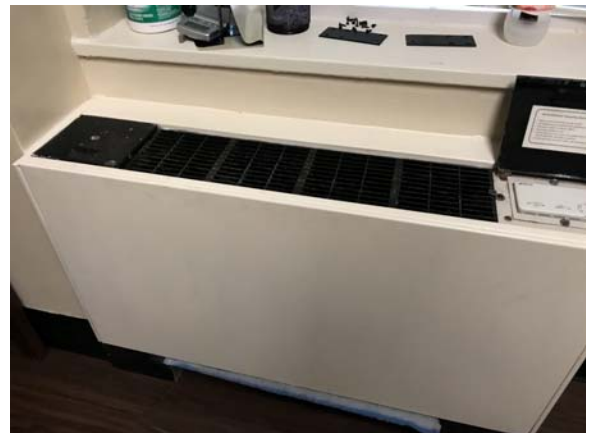
SLAY012e 5/12/2021 Console fan coil unit Room 147
