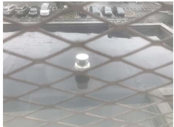
SLAY009e 5/12/2021 Centrifugal rooftop exhaust fan Lower roof
