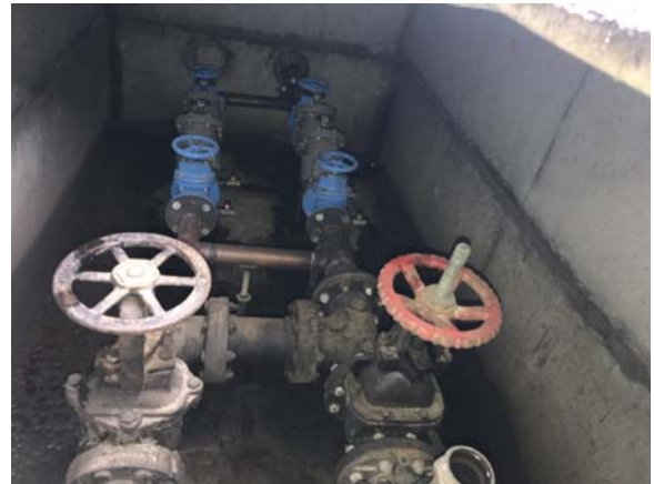
SLAY035e 5/12/2021 Domestic cold water backflow preventers Exterior
