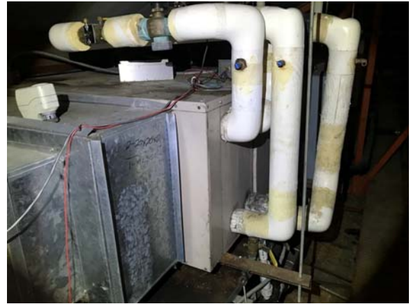
SLAY001e 5/12/2021 Fan coil unit Attic
