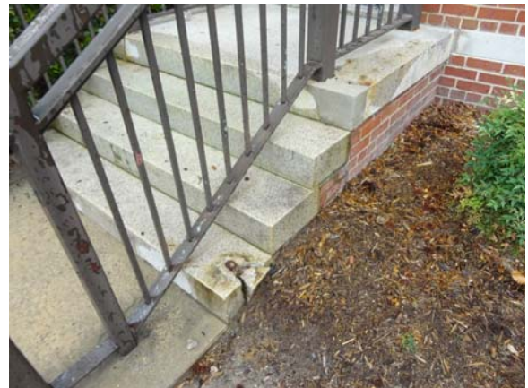
SLAY043a 5/12/2021 Granite steps with some failed repairs Southwest corner elevation
