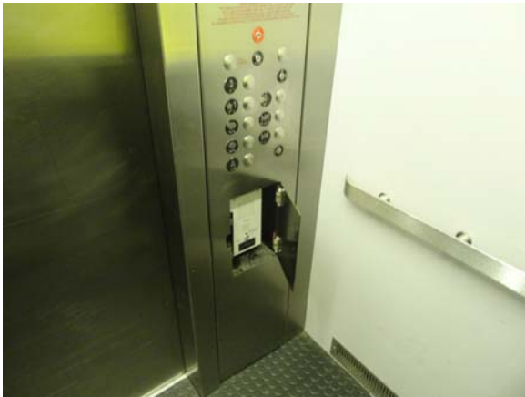
SLAY002a 5/12/2021 Accessible communication unit in non-ADA phone box Passenger elevator cab
