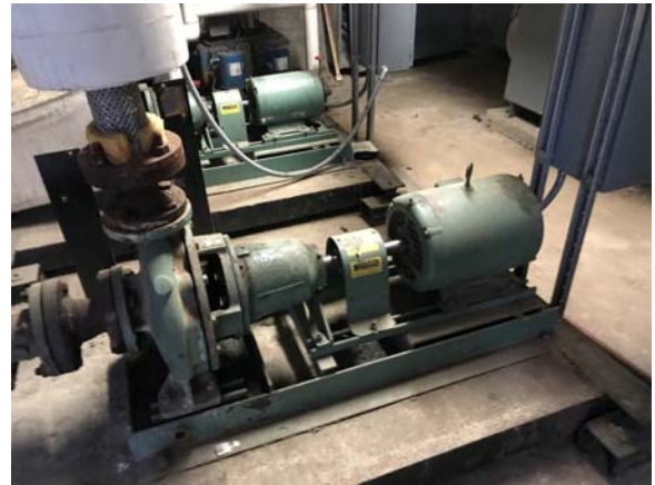
SLAY020e 5/12/2021 Heating hot water pumps Room 114E
