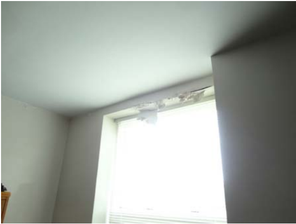
SLAY019a 5/12/2021 Ceiling damage possibly due to integral gutter issues Third floor
