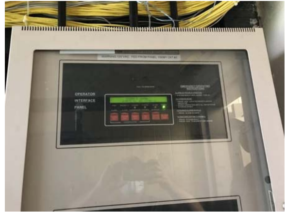
SLAY019e 5/12/2021 Main fire alarm panel Room 137
