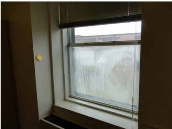
SLAY033a 5/12/2021 Window fogging issues First floor
