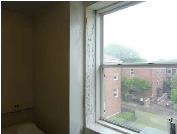
SLAY022a 5/12/2021 Water damage around exterior glazing Third floor
