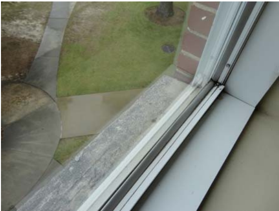
SLAY005a 5/12/2021 Aging metal-framed windows Third floor
