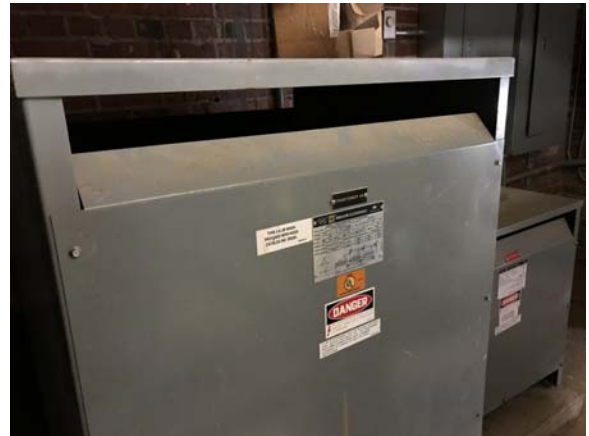
SLAY023e 5/12/2021 Step-down transformer Room 114E
