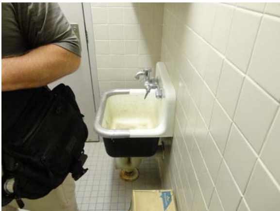
SLAY018a 5/12/2021 Wall-mounted service sink Third floor, janitor's closet
