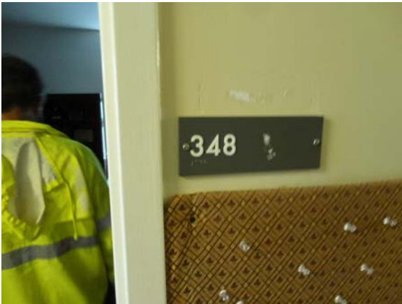
SLAY008a 5/12/2021 Accessible room signage but damaged wall paint Third floor corridor
