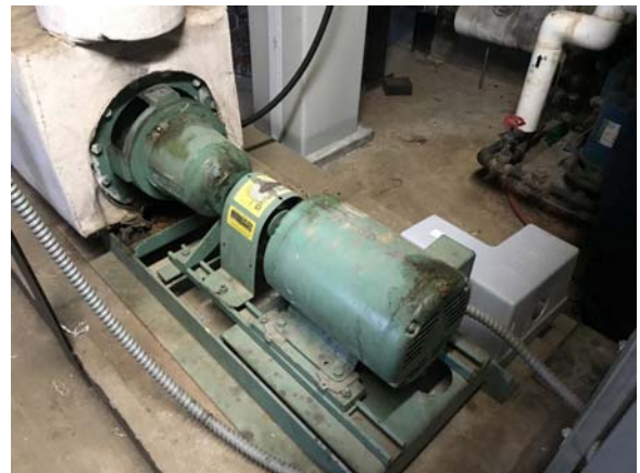
SLAY021e 5/12/2021 Chilled water pump Room 114E
