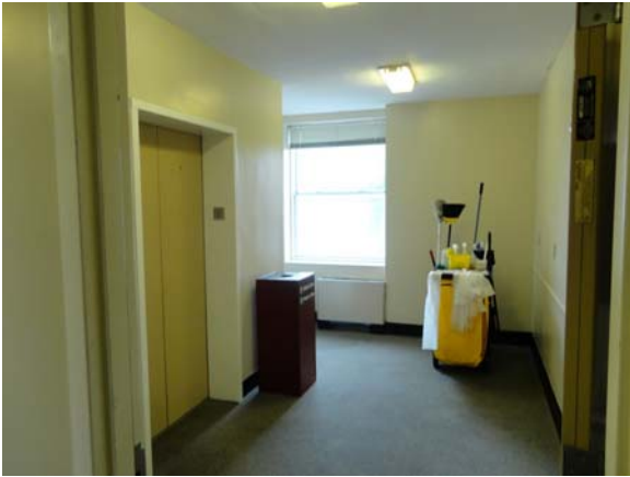
SLAY004a 5/12/2021 Worn carpeting and older paint on walls and ceiling Third floor corridor
