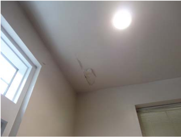
SLAY031a 5/12/2021 Unrepaired water damage to lobby ceiling First floor, entry lobby
