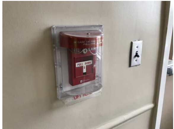
SLAY005e 5/12/2021 Manual pull fire alarm device Third floor corridor
