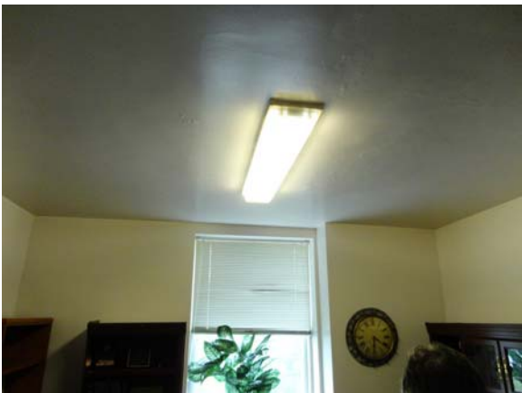
SLAY009a 5/12/2021 Some finish damage on painted ceiling Third floor, office
