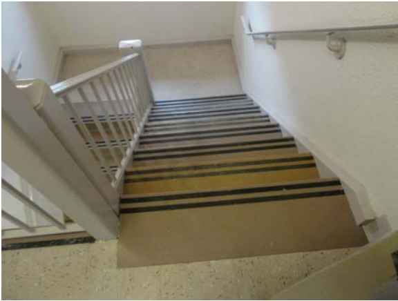
SLAY007a 5/12/2021 Worn rubber stair treads Third floor, stair tower
