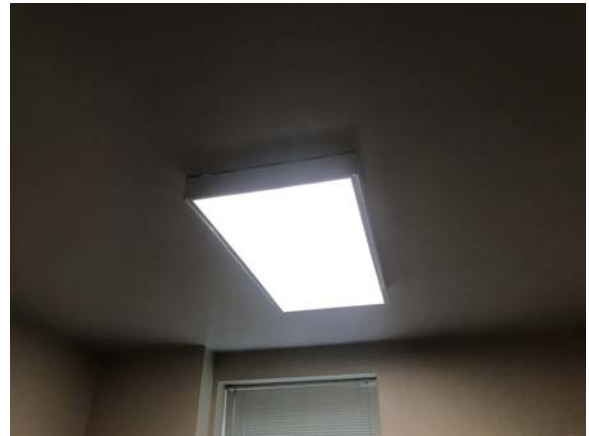
SLAY011e 5/12/2021 T8 troffer lighting fixture Room 147
