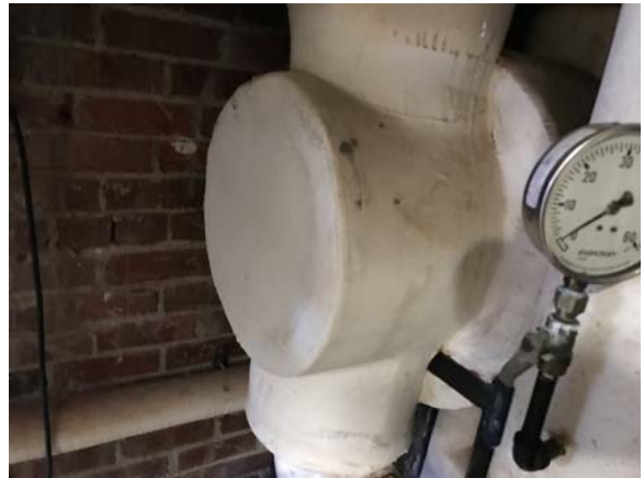
SLAY026e 5/12/2021 Shell-and-tube heat exchanger Room 114E
