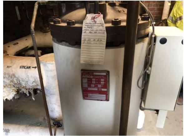
SLAY028e 5/12/2021 Domestic hot water heater exchanger Room 114E
