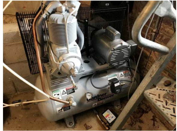
SLAY031e 5/12/2021 Controls air compressor Room 114E
