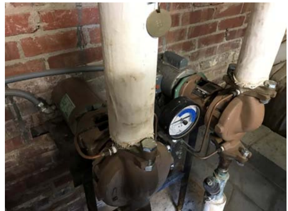
SLAY030e 5/12/2021 Domestic hot water pumps Room 114E
