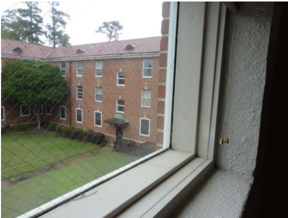
SLAY023a 5/12/2021 Original single-pane wire glass stair tower window Third floor, stair tower
