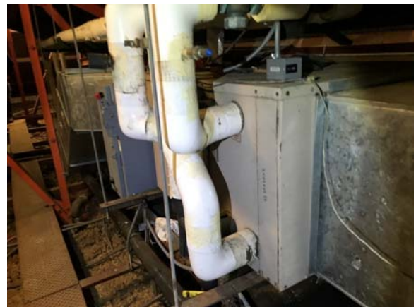
SLAY003e 5/12/2021 Fan coil unit Attic
