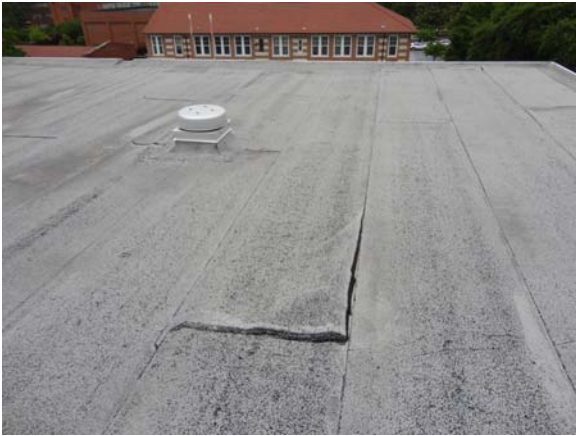
SPEI004a 5/11/2021 Blistered cap sheet Upper main roof
