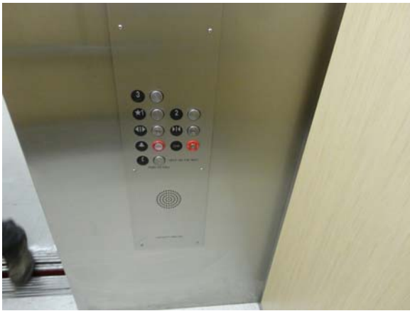
SPEI001a 5/11/2021 Accessible elevation control panel Passenger elevator cab
