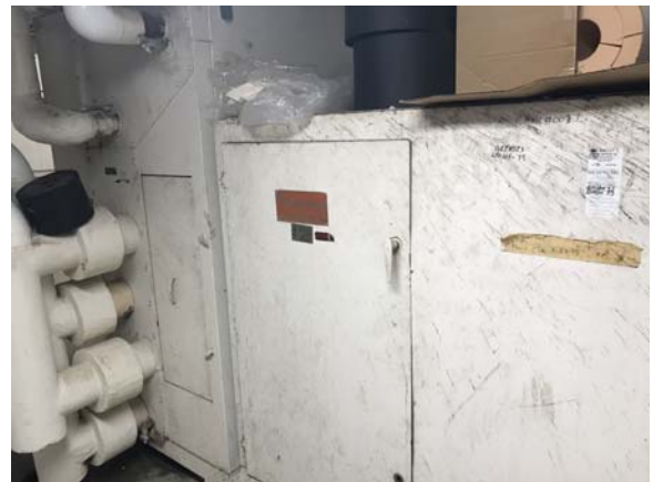
SPEI033e 5/11/2021 Air handling unit AHU-001 Room 165
