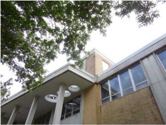
SPEI046a 5/11/2021 Upper masonry step cracking Northwest upper corner of third floor
