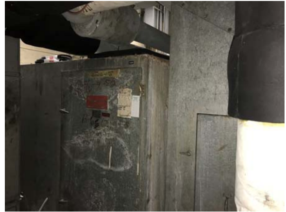
SPEI019e 5/11/2021 Air handling unit AHU-002 Room 160
