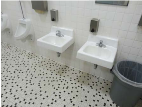
SPEI025a 5/11/2021 Partially accessible lavatories Second floor, men's restroom
