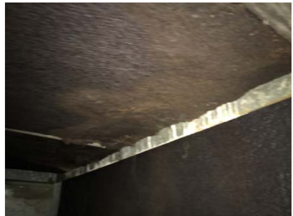
SPEI021e 5/11/2021 Insulation spalling inside AHU-002 Room 160
