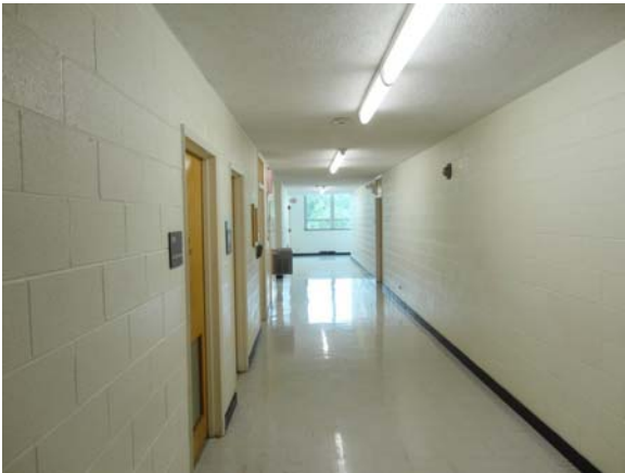
SPEI017a 5/11/2021 Original 9x9 vinyl flooring and original textured ceiling Third floor corridor
