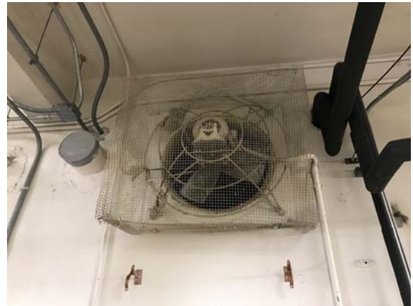
SPEI044e 5/11/2021 Propeller-style exhaust fan with louvers Room 165
