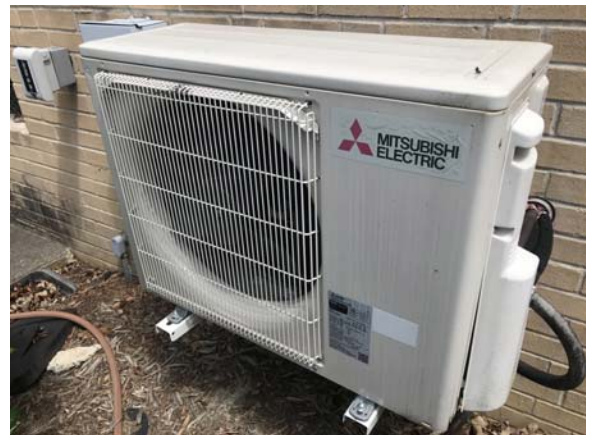
SPEI045e 5/11/2021 Ductless split condensing unit Site
