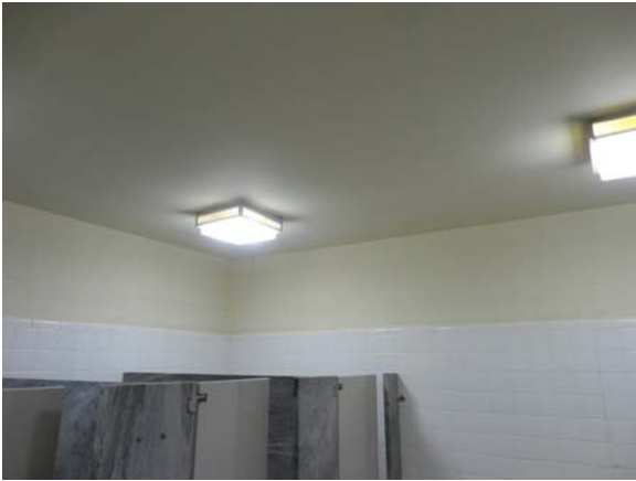
SPEI031a 5/11/2021 Painted ceiling Second floor, women's restroom
