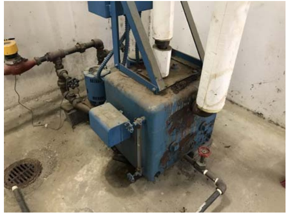
SPEI040e 5/11/2021 Condensate receiver Room 165
