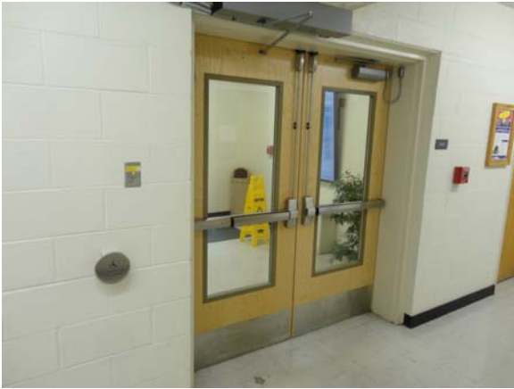
SPEI037a 5/11/2021 Upgraded stair access doors with power door assist First floor, stair tower
