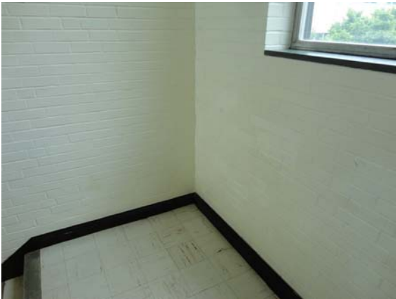
SPEI035a 5/11/2021 Signs of repaired stress cracks in corner of stair tower Second floor, stair tower
