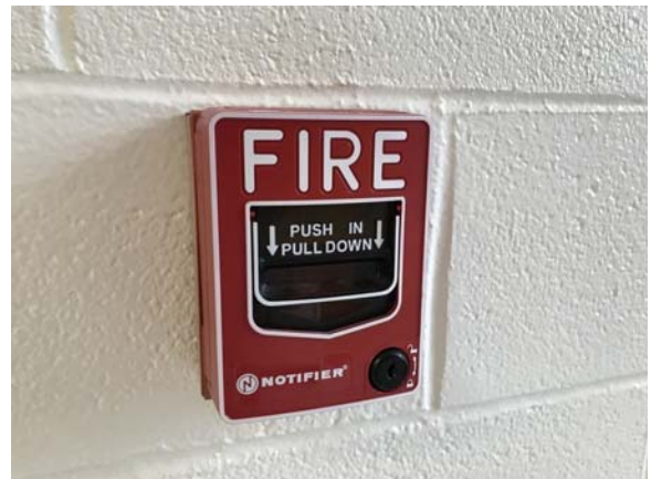
SPEI006e 5/11/2021 Manual pull fire alarm device Third floor corridor
