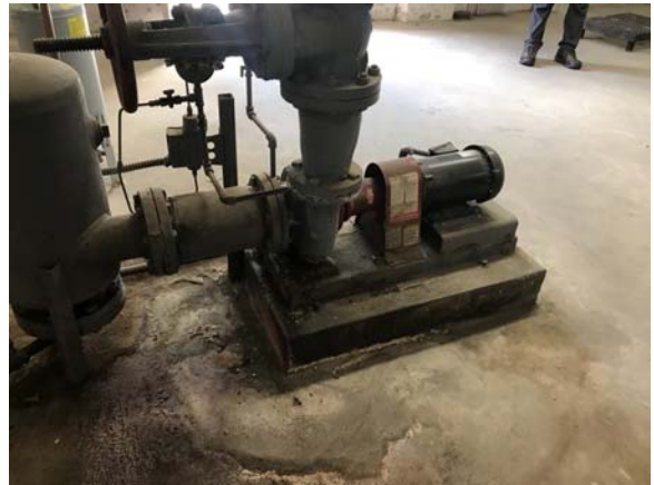
SPEI038e 5/11/2021 Heating hot water pump Room 165
