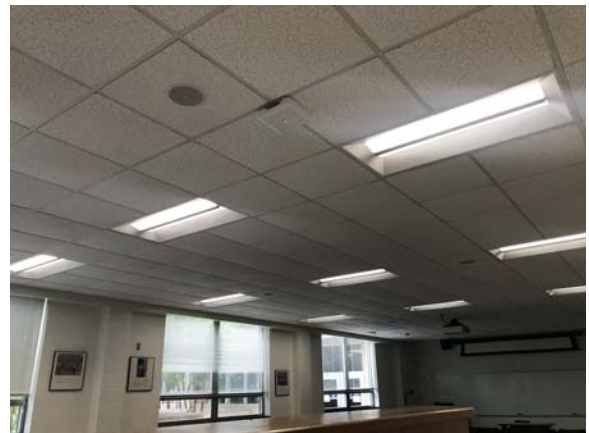
SPEI018e 5/11/2021 Recessed LED lighting fixtures Room 129
