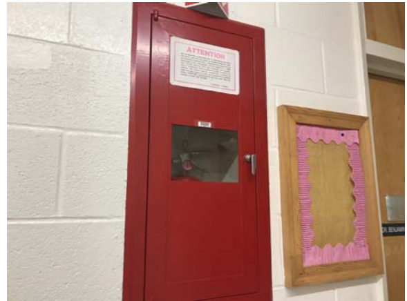
SPEI017e 5/11/2021 Fire extinguisher and suppression stand pipe Second floor corridor
