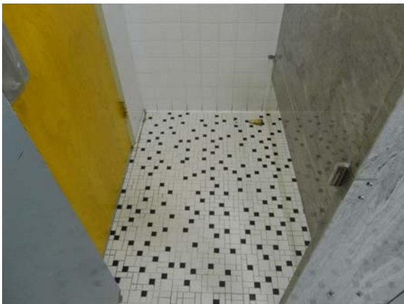
SPEI024a 5/11/2021 Narrow access at restroom entry Second floor, men's restroom
