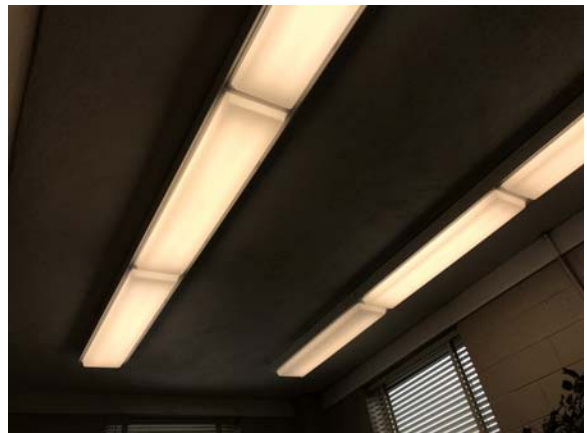
SPEI012e 5/11/2021 Retrofitted T8 lighting fixtures Third floor, office space
