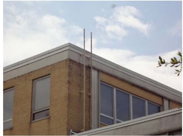
SPEI052a 5/11/2021 No safe guards on upper roof transition ladder Northeast corner
