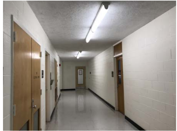
SPEI004e 5/11/2021 Retrofitted LED lighting fixtures Third floor corridor
