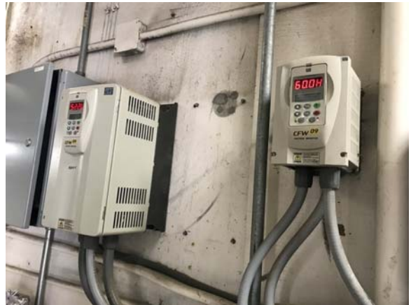
SPEI041e 5/11/2021 VFDs for AHU-001 and heating hot water pump Room 165
