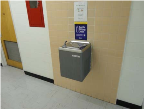
SPEI019a 5/11/2021 Older nonaccessible single-level water fountain Third floor corridor
