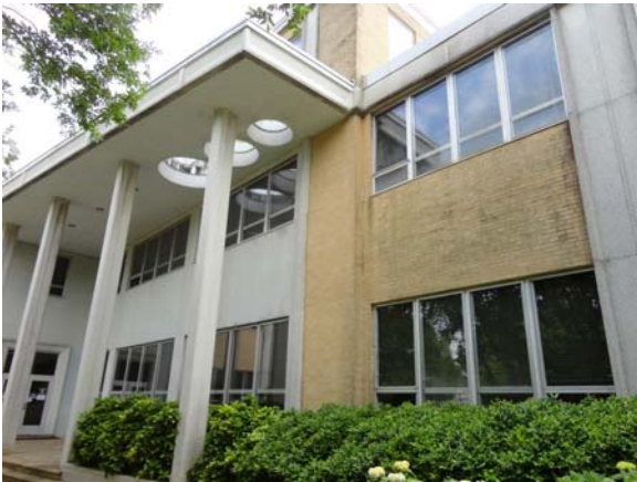
SPEI047a 5/11/2021 Stained exterior masonry and precast concrete panels Northwest elevation
