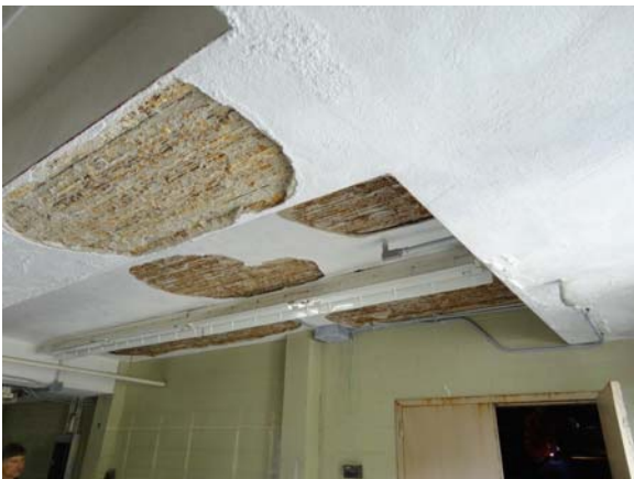
SPEI061a 5/11/2021 Heavy spalling on textured ceiling Basement, mechanical area
