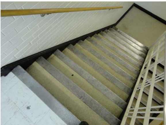
SPEI009a 5/11/2021 Worn stair treads Third floor, stair tower
