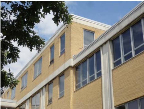
SPEI059a 5/11/2021 Upper masonry step cracking Southwest upper corner of third floor
