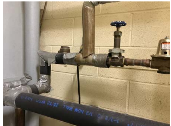
SPEI009e 5/11/2021 Insulated copper supply piping Room 319
