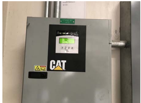
SPEI027e 5/11/2021 Automatic transfer switch Room 165
