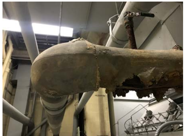
SPEI015e 5/11/2021 Suspect asbestos insulation Room 252
