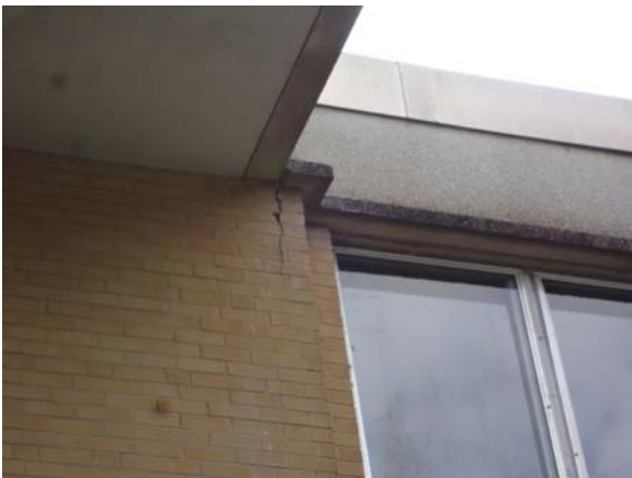
SPEI049a 5/11/2021 Vertical stress cracks on north elevation Northwest upper corner of third floor
