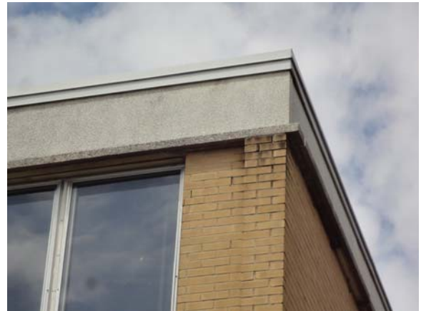
SPEI054a 5/11/2021 Upper corner masonry step cracking Southeast upper corner of third floor
