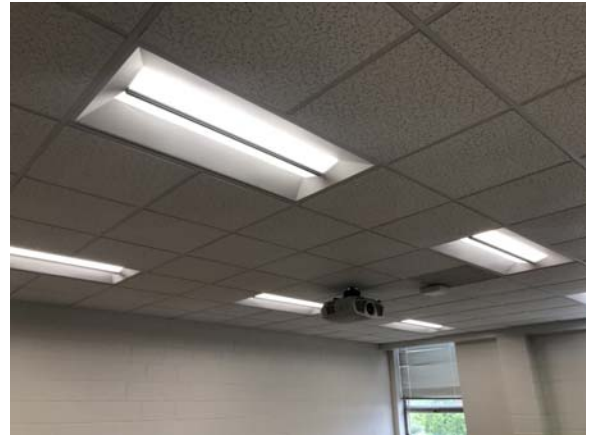
SPEI007e 5/11/2021 Recessed LED lighting fixtures Room 306
