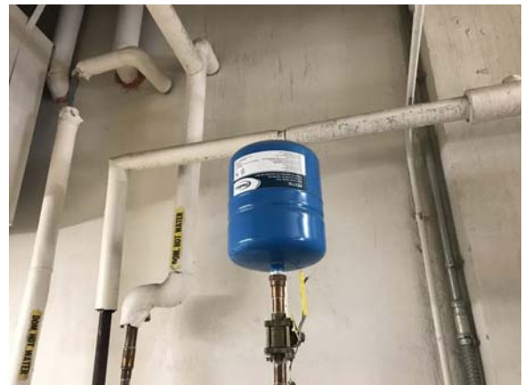
SPEI036e 5/11/2021 Expansion tank Room 165
