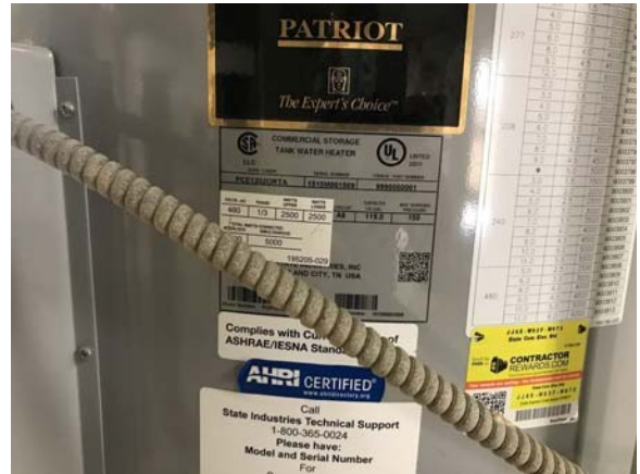
SPEI035e 5/11/2021 Residential electric water heater Room 165
