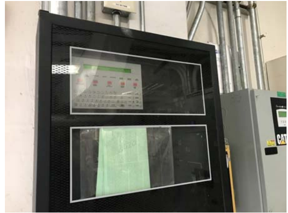
SPEI025e 5/11/2021 Main fire alarm panel Room 165
