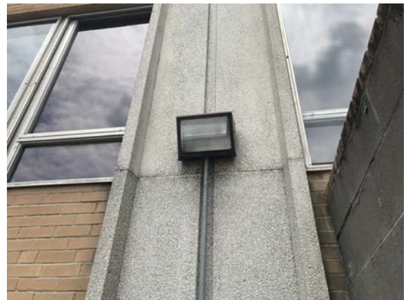
SPEI024e 5/11/2021 HID wallpack Exterior
