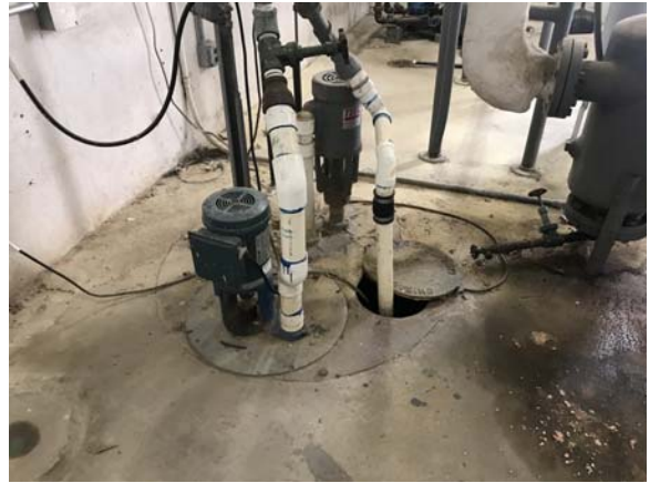
SPEI037e 5/11/2021 Sump pump Room 165
