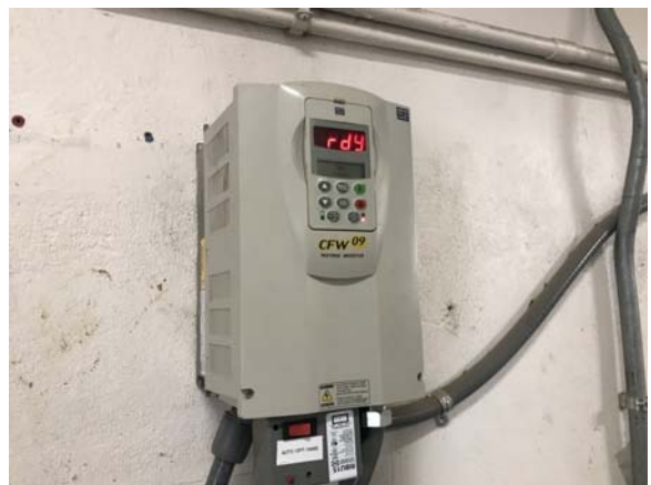
SPEI042e 5/11/2021 VFD for chilled water pump Room 165
