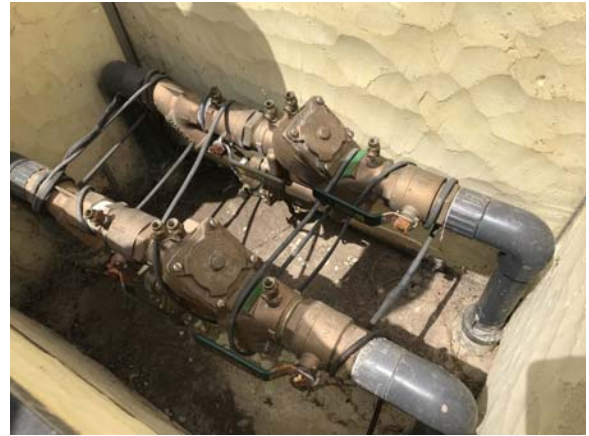
SPEI046e 5/11/2021 Backflow preventers for water main Exterior
