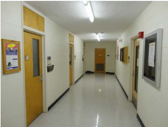
SPEI038a 5/11/2021 Original 9x9 vinyl flooring and original textured ceiling First floor corridor
