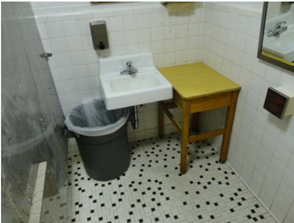
SPEI041a 5/11/2021 Partially accessible wall-hung lavatory and power door assist First floor, all-gender restroom
