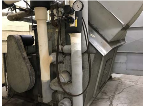
SPEI013e 5/11/2021 Air handling unit AHU-003 Room 252
