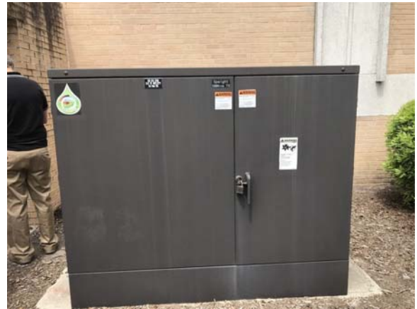
SPEI023e 5/11/2021 Oil-filled transformer Exterior
