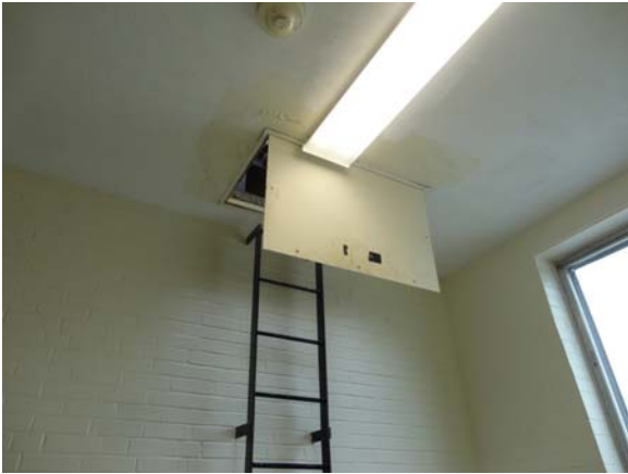
SPEI007a 5/11/2021 Aging original lower roof hatch Third floor, stair tower
