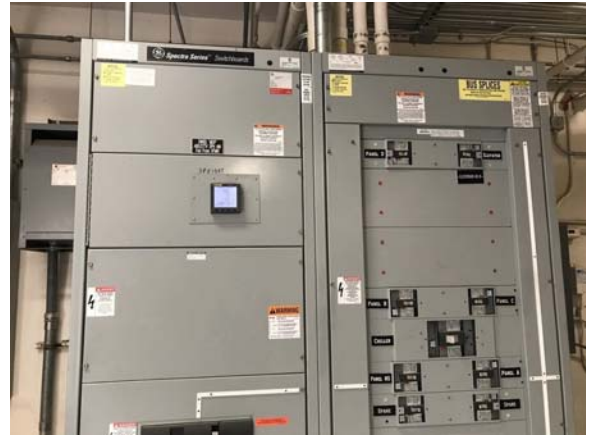
SPEI028e 5/11/2021 Main switchboard Room 165
