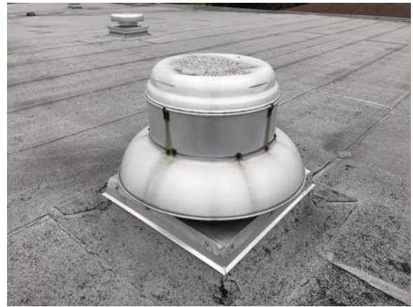
SPEI001e 5/11/2021 Centrifugal rooftop exhaust fan Roof
