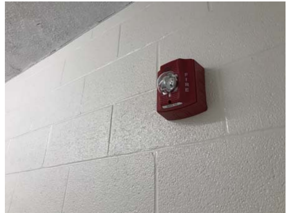
SPEI005e 5/11/2021 Horn with strobe fire alarm device Third floor corridor
