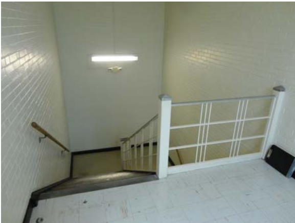
SPEI008a 5/11/2021 Nonaccessible inner and outer stair rails Third floor, stair tower
