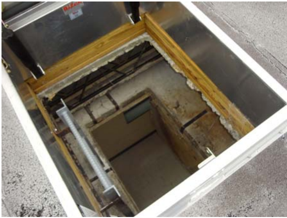
SPEI002a 5/11/2021 Poor lower hatch and no stair rail extension Roof hatch
