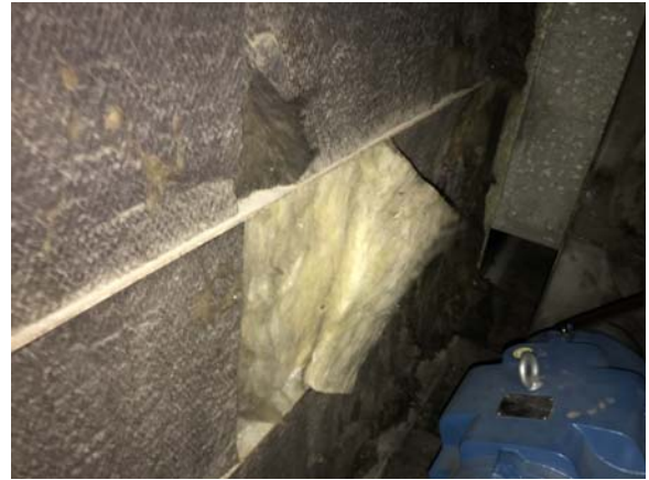
SPEI034e 5/11/2021 Insulation spalling inside AHU-001 Room 165
