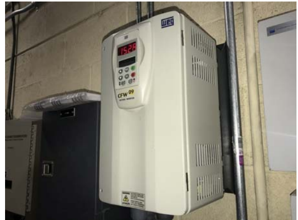
SPEI020e 5/11/2021 VFD for AHU-002 Room 160
