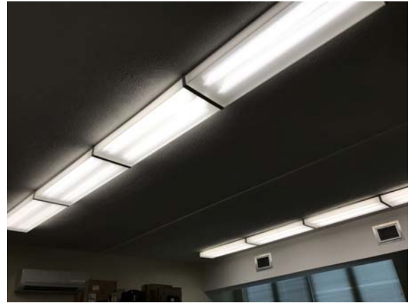
SPEI016e 5/11/2021 Retrofitted LED lighting fixtures Room 228
