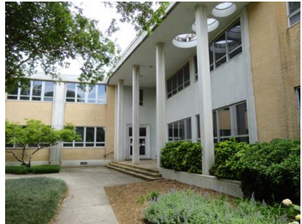
SPEI048a 5/11/2021 Lack of handrails at front entry steps Northwest elevation
