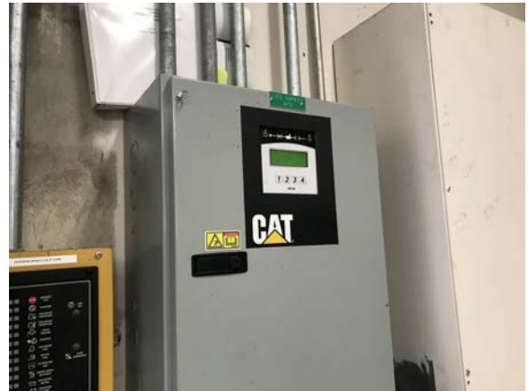
SPEI026e 5/11/2021 Automatic transfer switch Room 165
