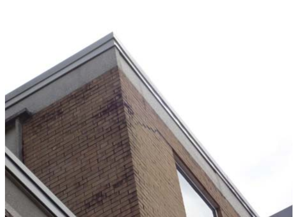
SPEI050a 5/11/2021 Step cracking on north elevation Northwest upper corner of third floor
