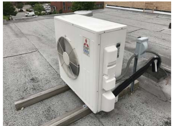
SPEI003e 5/11/2021 Ductless split condensing unit Roof
