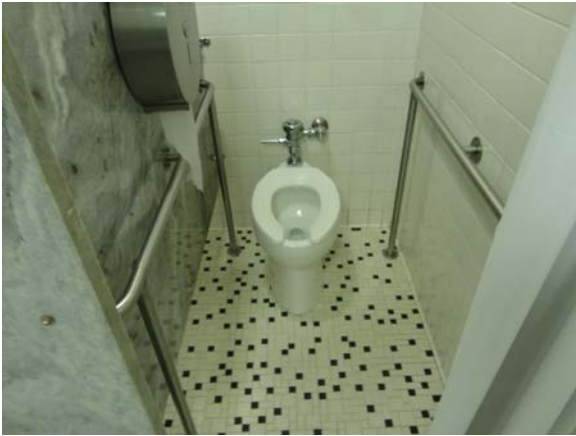
SPEI043a 5/11/2021 Partially accessible toilet stall First floor, restroom
