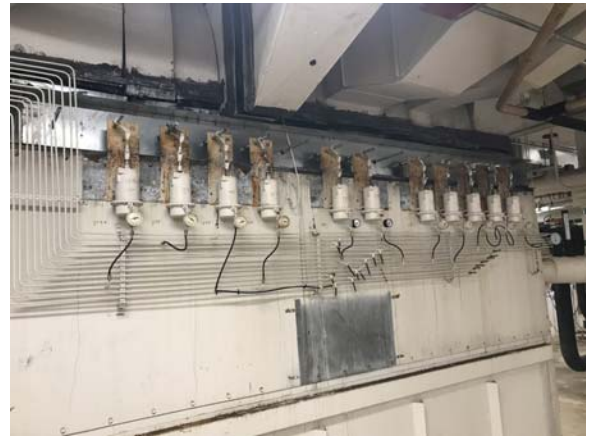
SPEI032e 5/11/2021 Zoned deck on AHU-001 Room 165
