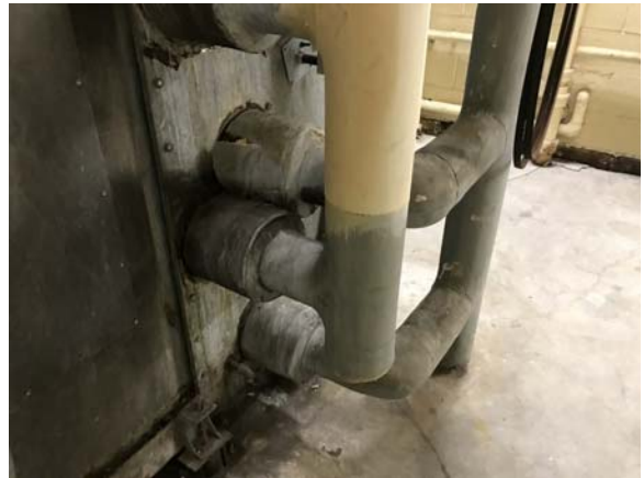
SPEI014e 5/11/2021 Suspect asbestos insulation Room 252
