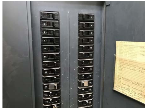
SPEI008e 5/11/2021 Local panelboard Room 318
