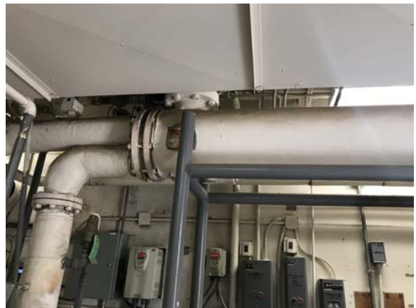
SPEI039e 5/11/2021 Heating hot water shell-and-tube heat exchanger Room 165
