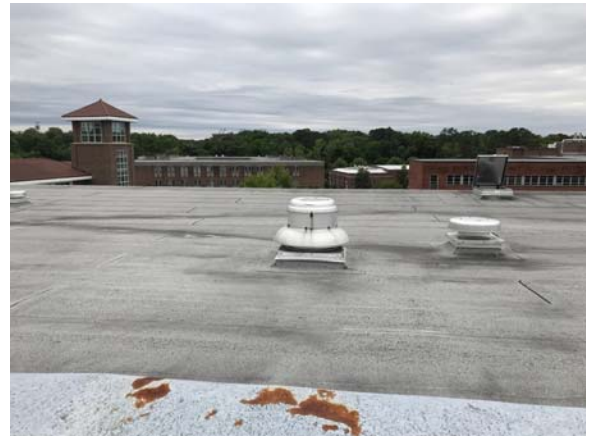
SPEI002e 5/11/2021 Centrifugal rooftop exhaust fan Roof
