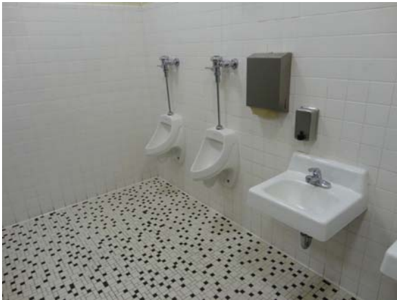
SPEI026a 5/11/2021 Partially accessible urinals Second floor, men's restroom
