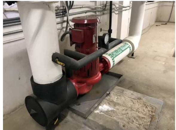
SPEI029e 5/11/2021 Chilled water pump Room 165
