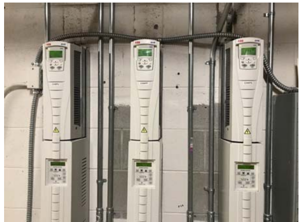
UMST021e 5/12/2021 VFDs for chilled water pumps Room 002
