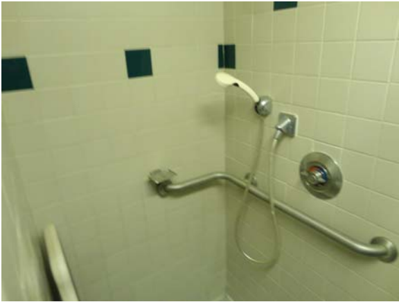
UMST025a 5/12/2021 Accessible roll-in shower Third floor, women's west hall bath
