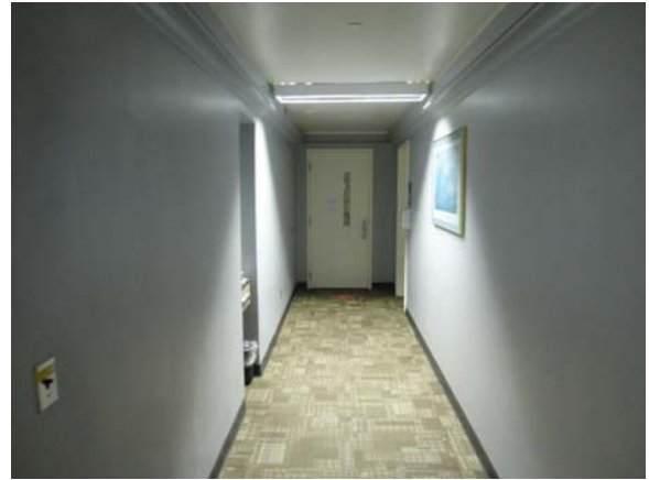
UMST044a 5/12/2021 Worn carpeting and painted walls and ceiling First floor, northeast corridor
