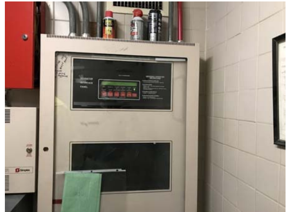
UMST014e 5/12/2021 Main fire alarm panel Room 108
