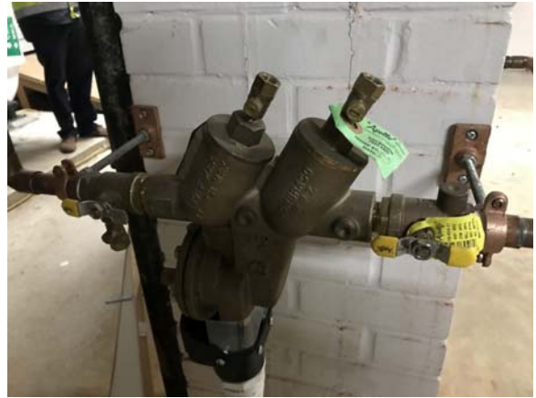
UMST022e 5/12/2021 Backflow preventer for makeup water Room 002
