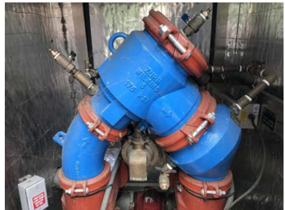
UMST036e 5/12/2021 Backflow preventer for fire suppression Exterior
