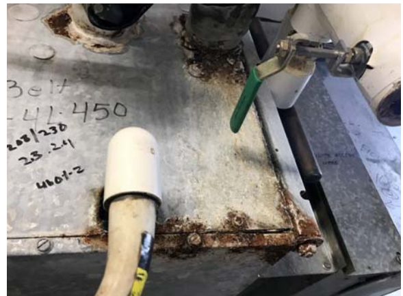
UMST033e 5/12/2021 Corrosion on fan coil unit Room 164
