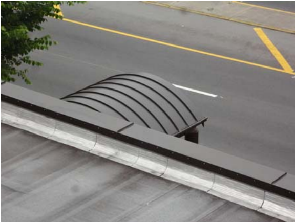
UMST007a 5/12/2021 One of two standing-seam barrel arch entry canopies South main entry
