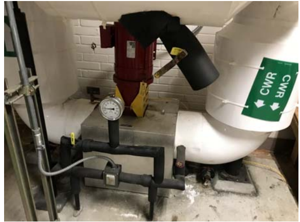
UMST016e 5/12/2021 Chilled water pump Room 002
