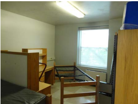
UMST012a 5/12/2021 Older VCT and painted walls and ceiling Third floor, dorm room
