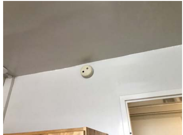
UMST008e 5/12/2021 Covered fire suppression sprinkling device Room 302
