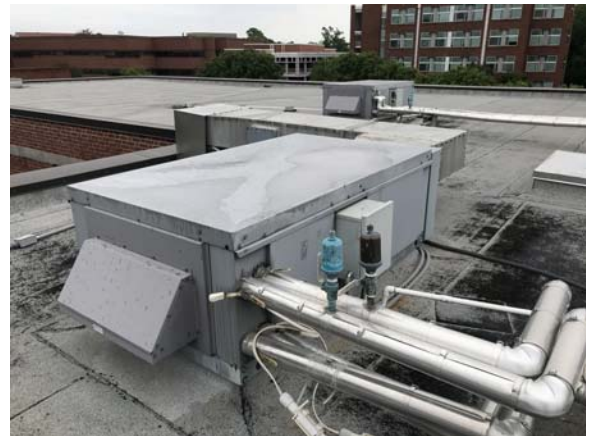
UMST003e 5/12/2021 Rooftop makeup air handling unit Roof
