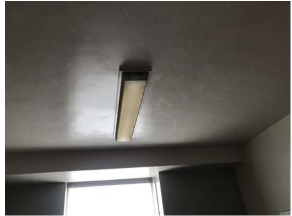
UMST007e 5/12/2021 T8 troffer lighting fixture Room 302
