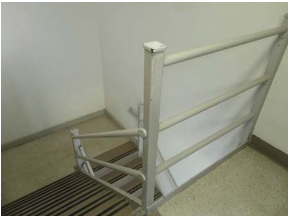
UMST009a 5/12/2021 Wide picket spacing on inner switchback railing Third floor, stair tower
