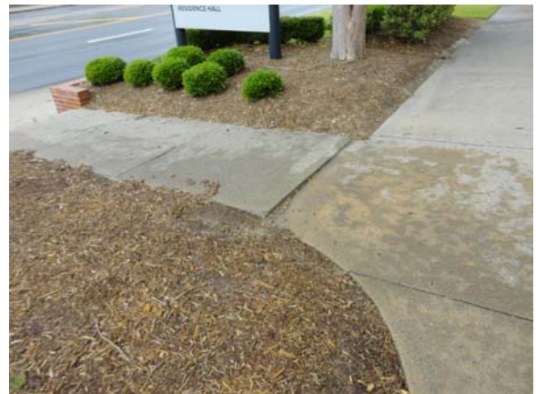
UMST048a 5/12/2021 Some differential settlement on concrete sidewalks Southeast corner of site
