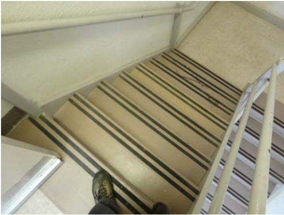
UMST031a 5/12/2021 Wear on the rubber stair treads Third floor, stair tower
