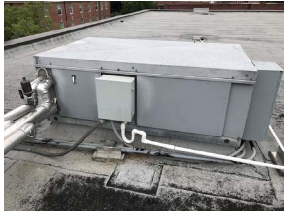
UMST005e 5/12/2021 Rooftop makeup air handling unit Roof
