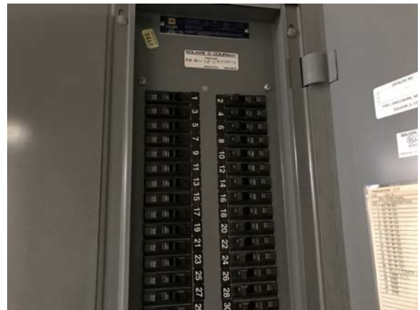
UMST012e 5/12/2021 Local panelboard Second floor corridor
