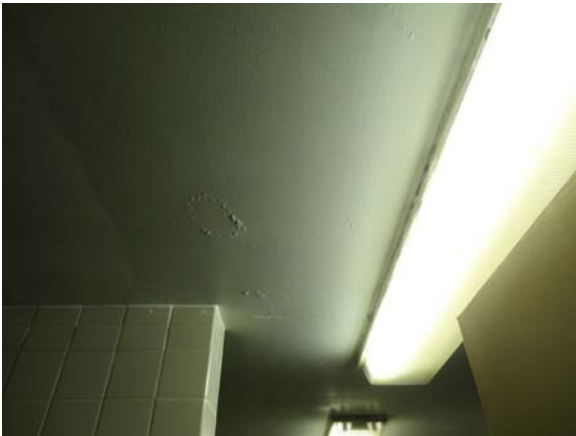
UMST026a 5/12/2021 Some localized painted ceiling damage Third floor, women's west hall bath
