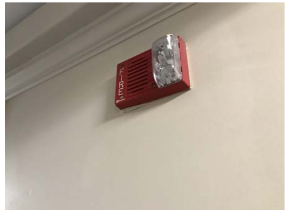
UMST009e 5/12/2021 Horn with strobe fire alarm device Third floor corridor
