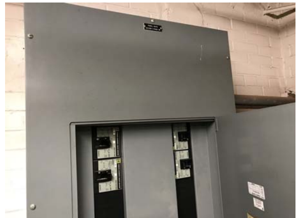
UMST027e 5/12/2021 Distribution panelboard Room 007
