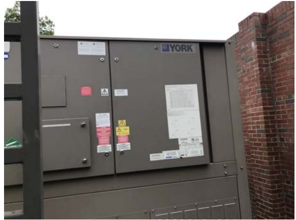
UMST028e 5/12/2021 Air-cooled packaged chiller Room 007
