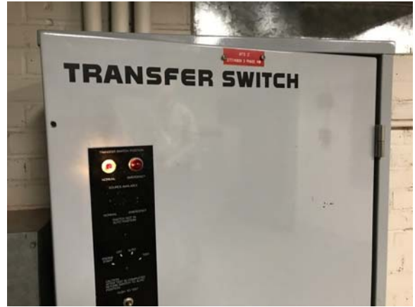
UMST025e 5/12/2021 Automatic transfer switch Room 007
