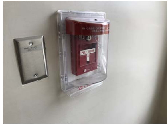
UMST010e 5/12/2021 Manual pull fire alarm device Third floor corridor
