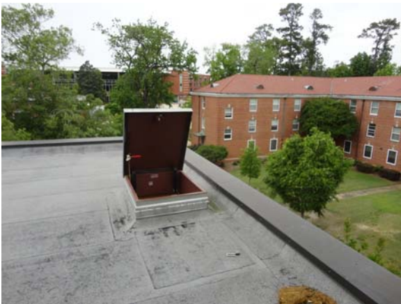
UMST003a 5/12/2021 One of three roof hatches located at edge of roof Roof
