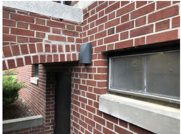
UMST023e 5/12/2021 LED sconce lighting fixture Southeast corner
