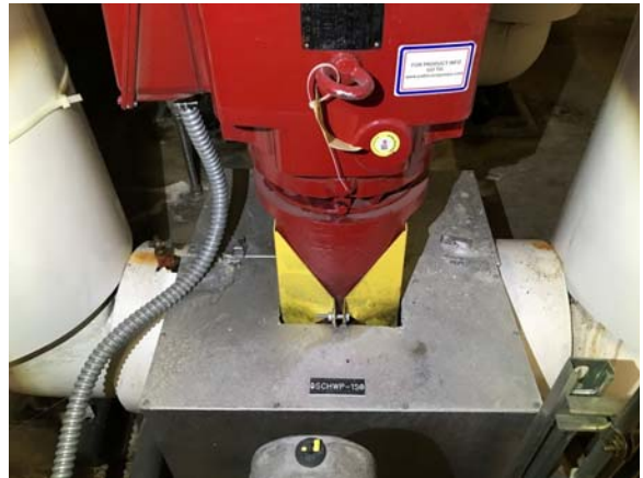
UMST020e 5/12/2021 Chilled water pump Room 002
