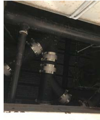
UMST013e 5/12/2021 Cast-iron drain piping with hubless connections Trash room
