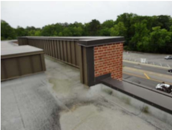
UMST005a 5/12/2021 Raised parapet cap at front elevation Upper center of south elevation
