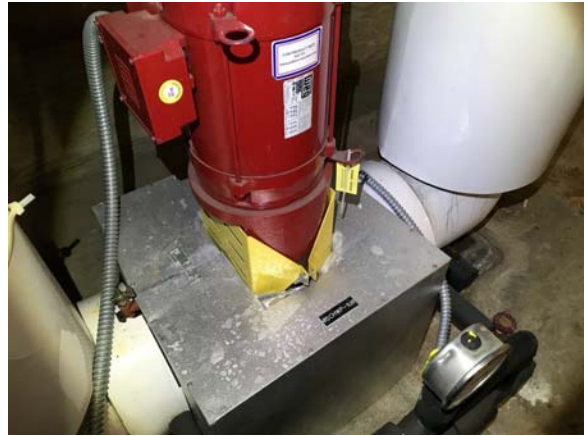
UMST019e 5/12/2021 Chilled water pump Room 002
