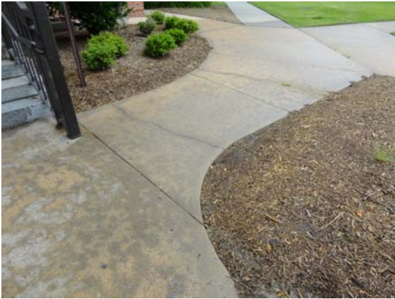
UMST049a 5/12/2021 Some differential settlement on concrete sidewalks Southeast corner of site
