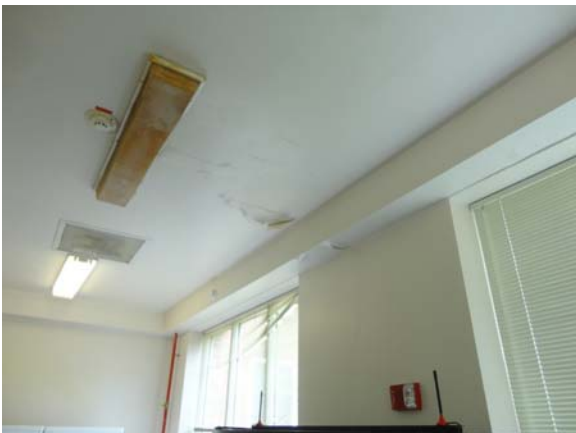
UMST065a 5/12/2021 Unrepaid water damage to painted ceiling First floor, south laundry
