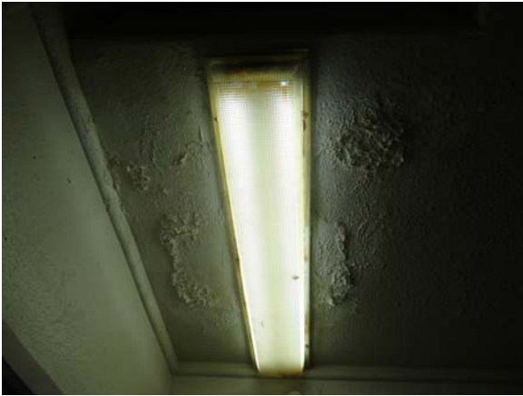
UMST028a 5/12/2021 Unrepared ceiling water damage at roof hatch Third floor, central stair tower
