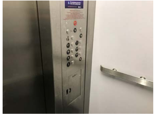
UMST001e 5/12/2021 Cab interior Elevator
