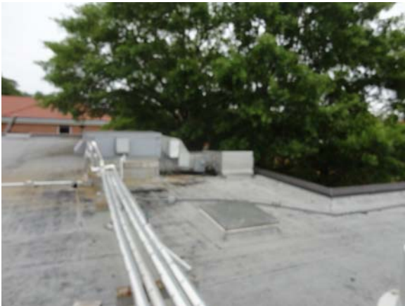
UMST008a 5/12/2021 Tree overhang over portion of main roof Main roof
