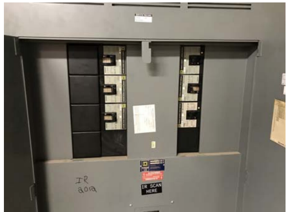
UMST024e 5/12/2021 Main distribution panelboard Room 007
