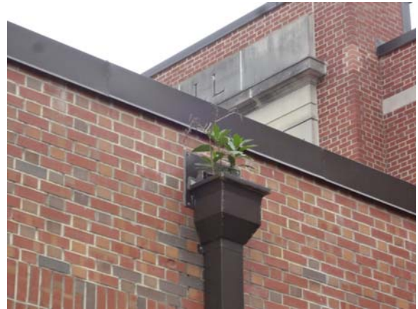
UMST052a 5/12/2021 Sign of blocked drain scupper Lower south roof
