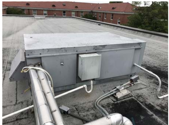
UMST006e 5/12/2021 Rooftop makeup air handling unit Roof
