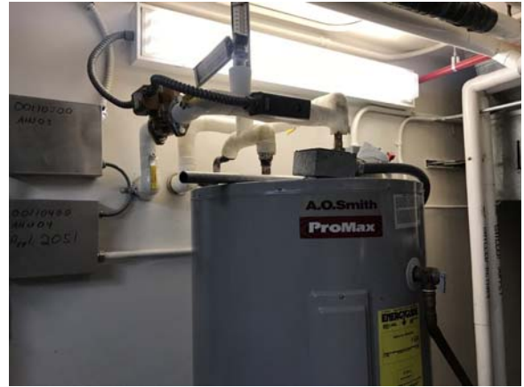
UMST031e 5/12/2021 Residential electric water heater Room 007
