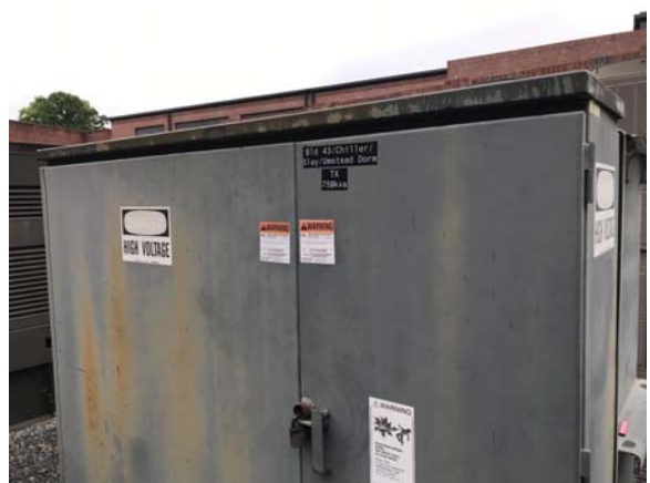
UMST029e 5/12/2021 Oil-filled transformer Room 007
