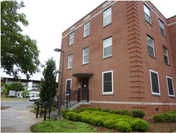
UMST055a 5/12/2021 Flanking handrails on egress stair Southwest wing
