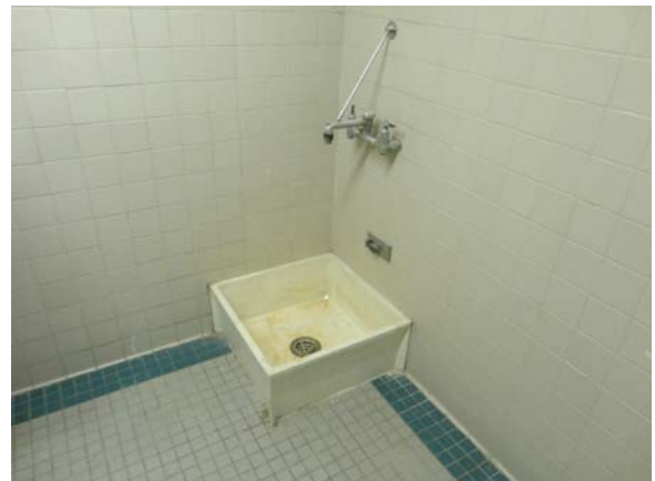
UMST042a 5/12/2021 Newer floor-mounted mop sink First floor, janitor's closet
