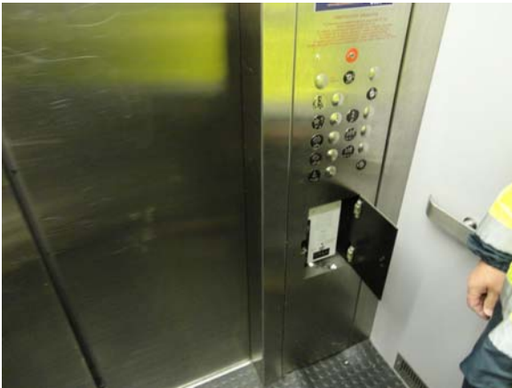
UMST002a 5/12/2021 Accessible two-way communication in non-ADA phone box Passenger elevator cab
