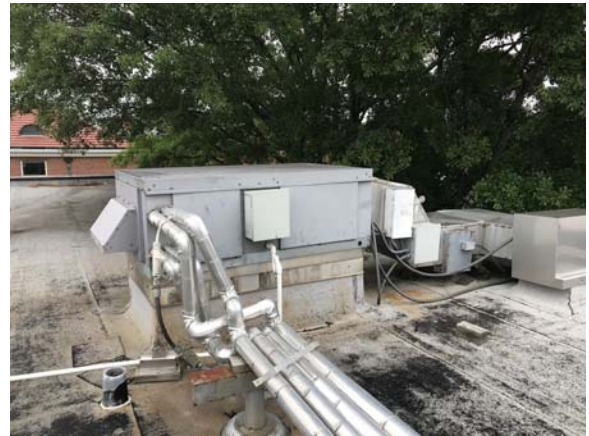
UMST002e 5/12/2021 Rooftop makeup air handling unit Roof
