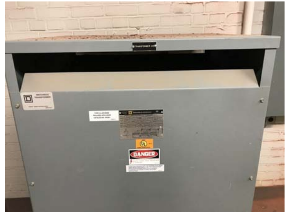
UMST026e 5/12/2021 Secondary step-down transformer Room 007
