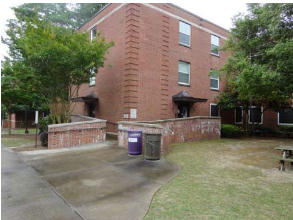
UMST059a 5/12/2021 Efflorescence on masonry site walls Central north wing
