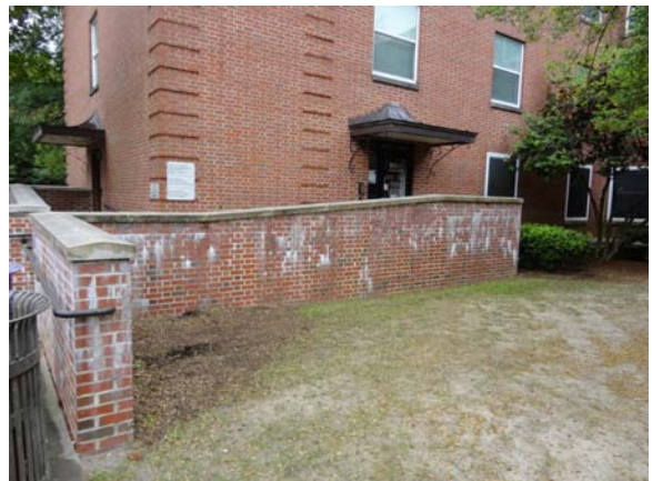
UMST060a 5/12/2021 Detail of heavy efflorescence Central north wing
