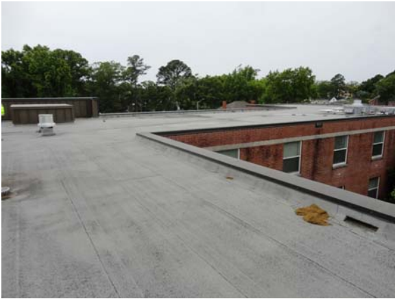
UMST004a 5/12/2021 Built-up roof with cap sheet and low parapet cap flashing Main flat roof
