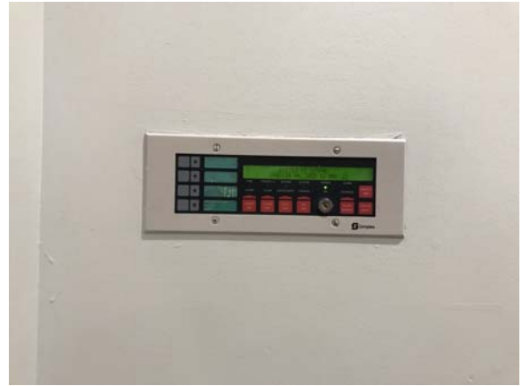
UMST034e 5/12/2021 Fire alarm annunciator panel Main lobby
