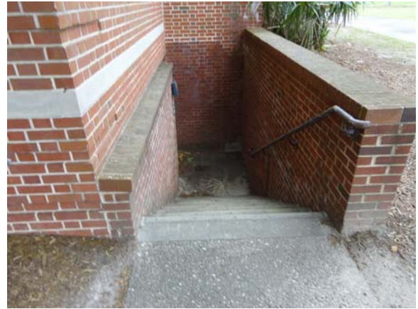
UMST062a 5/12/2021 Only one handrail on service stair East basement service entry
