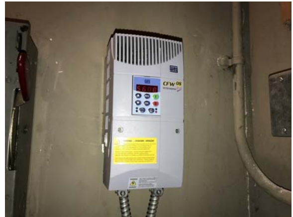
WHIC017e 5/10/2021 VFD for AHU-003 Room 118
