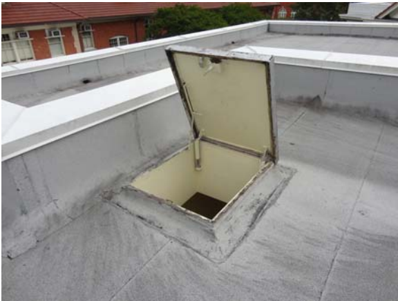
WHIC002a 5/10/2021 Deteriorated roof hatch Annex roof
