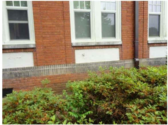
WHIC058a 5/10/2021 Peeling paint under windows Lower west elevation of original building
