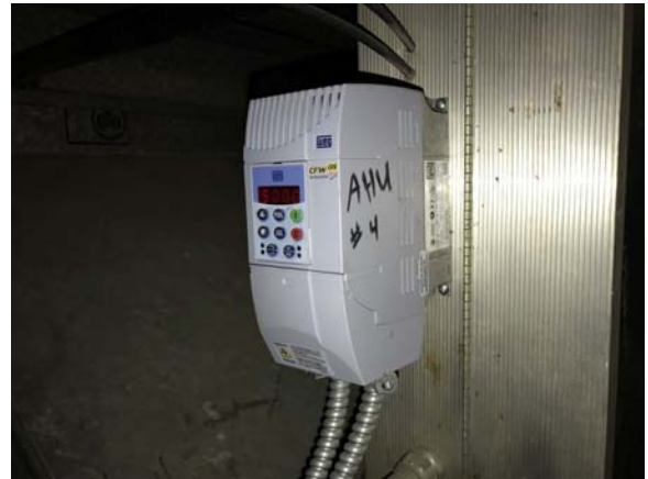
WHIC011e 5/10/2021 VFD for AHU-004 Room 214D
