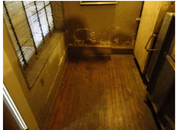
WHIC046a 5/10/2021 Badly deteriorated wood flooring First floor, mechanical room
