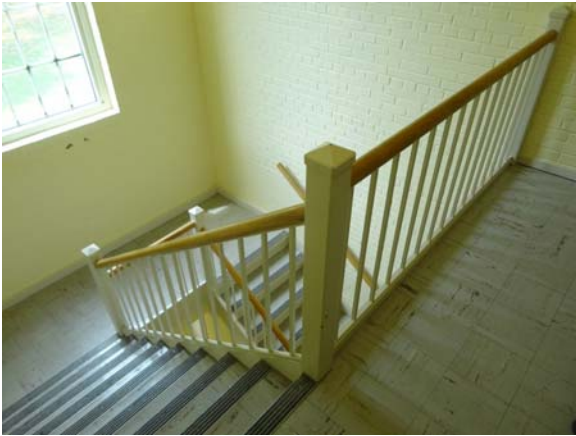
WHIC007a 5/10/2021 Low guardrail and inadequate switchback rail Second floor, annex stair tower
