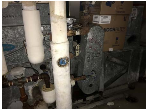
WHIC035e 5/10/2021 Air handling unit AHU-006 Room 117D
