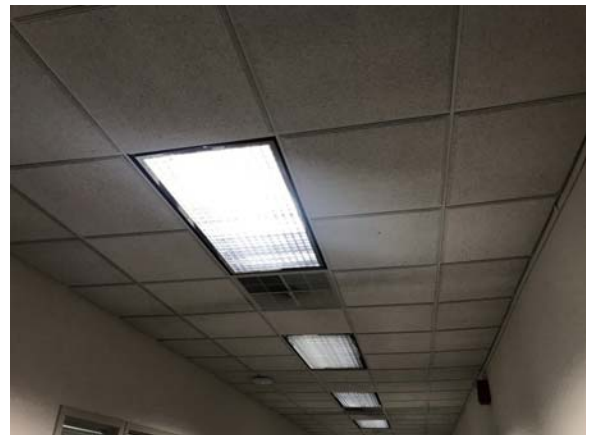
WHIC015e 5/10/2021 Retrofitted recessed T8 lighting fixtures First floor corridor
