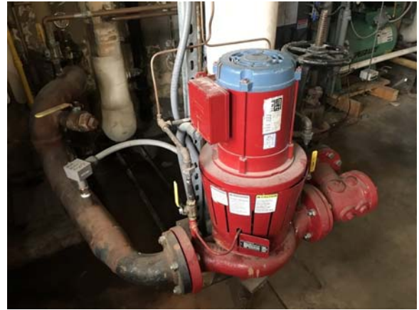
WHIC025e 5/10/2021 Heating hot water pump Room 117D
