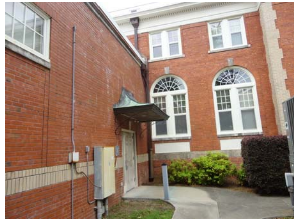
WHIC064a 5/10/2021 Entry doors and copper clad canopy North elevation of east wing
