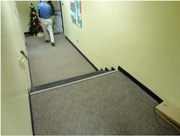
WHIC049a 5/10/2021 Inadequate handrails on corridor steps First floor, north annex corridor
