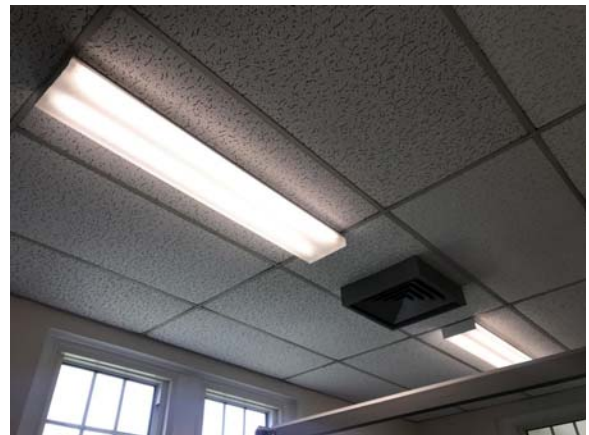
WHIC018e 5/10/2021 Retrofitted T8 troffer lighting fixture Room 106K
