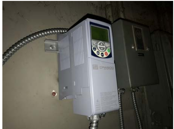
WHIC023e 5/10/2021 VFD for AHU-001 Room 119A
