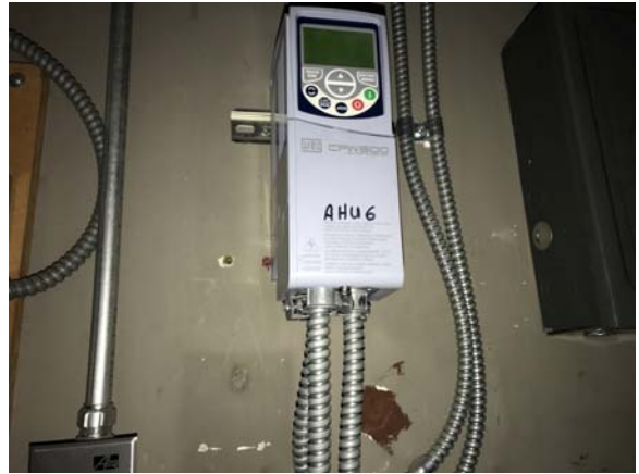
WHIC034e 5/10/2021 VFD for AHU-006 Room 117D
