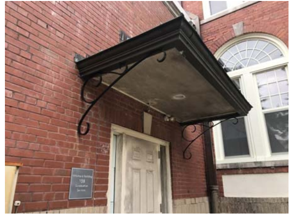
WHIC040e 5/10/2021 Recessed LED lighting fixture Exterior soffit
