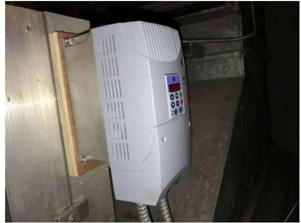
WHIC013e 5/10/2021 VFD for AHU-005 Room 214D
