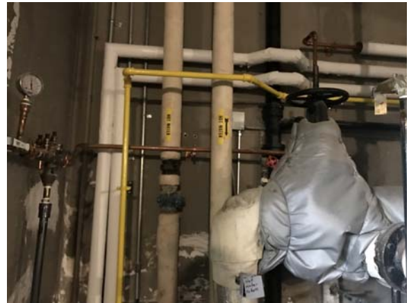
WHIC026e 5/10/2021 Potential asbestos piping Room 117D
