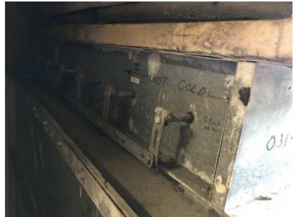
WHIC002e 5/10/2021 Zoned deck for AHU-002 Room 227
