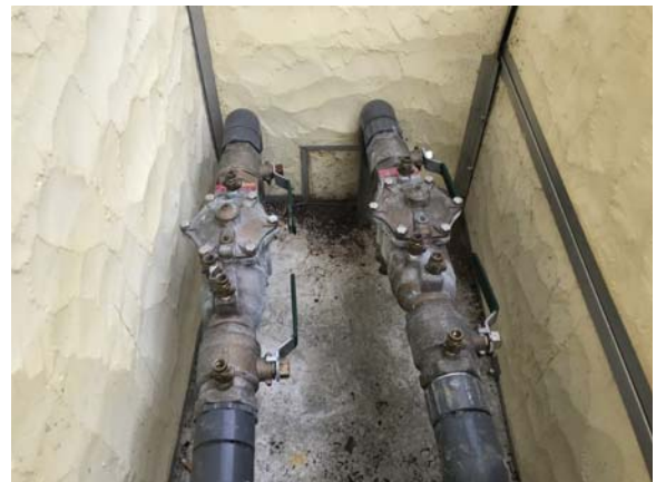
WHIC042e 5/10/2021 Backflow preventers for water main Site
