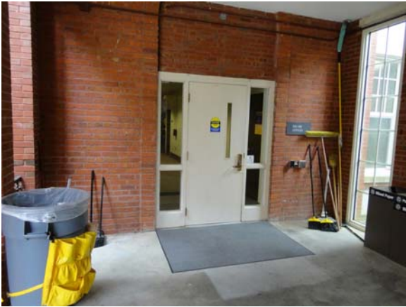
WHIC067a 5/10/2021 Newer hollow-metal door with sidelights and power assist First floor, north entry to original building
