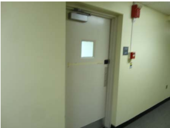
WHIC012a 5/10/2021 No positive latching hardware on stair tower door Second floor, stair tower
