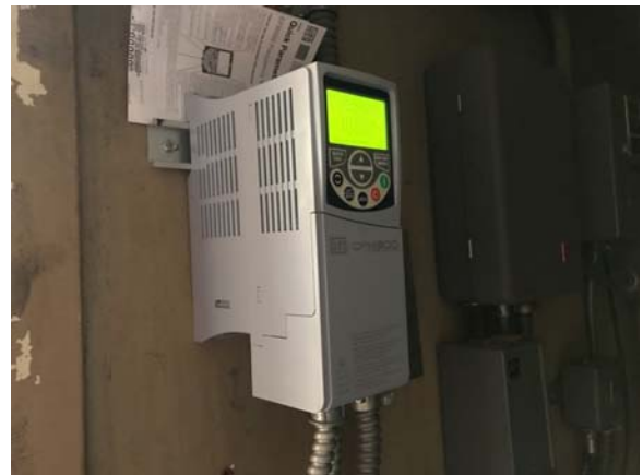
WHIC003e 5/10/2021 VFD for AHU-002 Room 227
