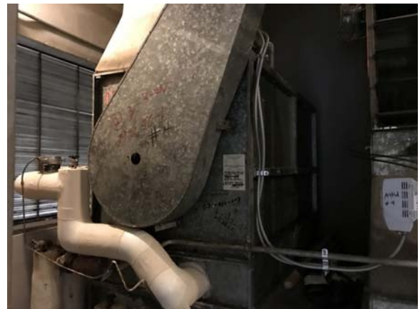
WHIC009e 5/10/2021 Air handling unit AHU-004 Room 214D
