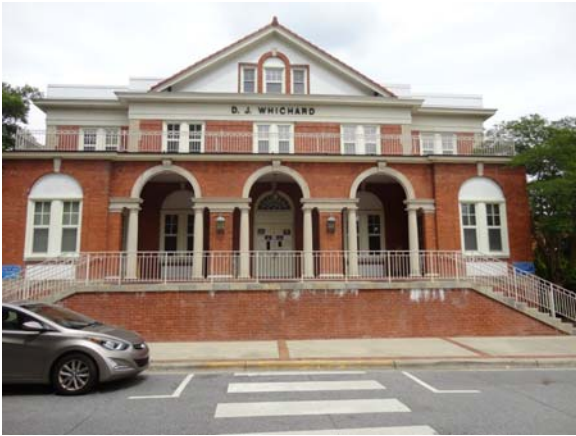
WHIC061a 5/10/2021 Signs of efflorescence on entry steps South elevation of original building
