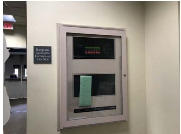
WHIC020e 5/10/2021 Main fire alarm panel First floor corridor
