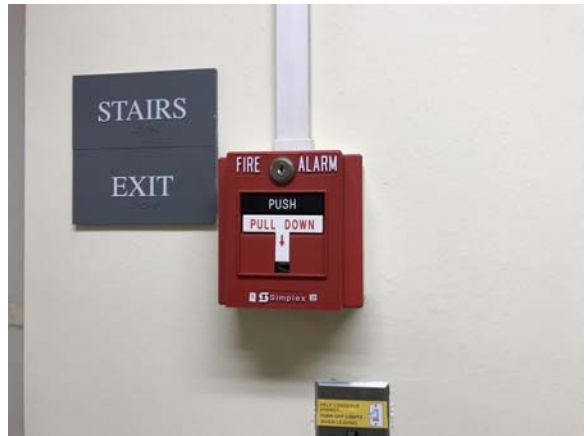
WHIC006e 5/10/2021 Manual pull fire alarm device Second floor corridor
