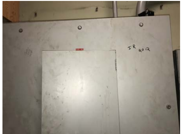
WHIC038e 5/10/2021 Main distribution panelboard Room 119
