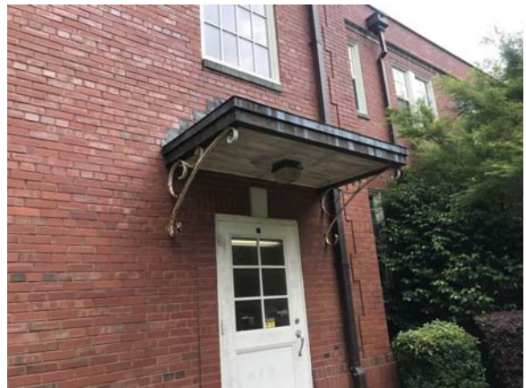
WHIC024e 5/10/2021 Ceiling-mounted HID lighting fixture Exterior soffit
