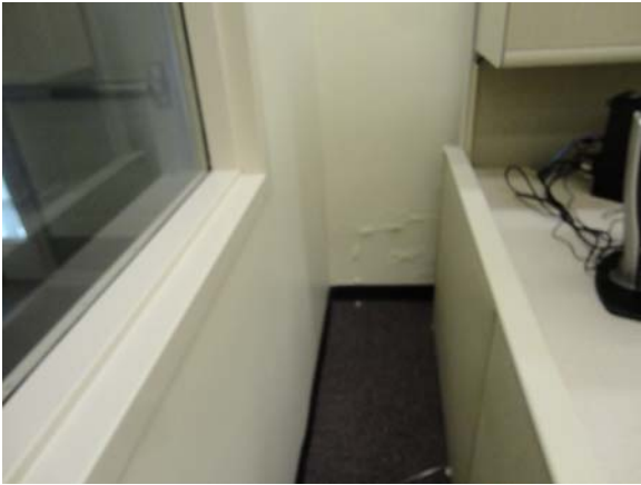
WHIC034a 5/10/2021 More localized signs of water infiltration First floor, east wing addition
