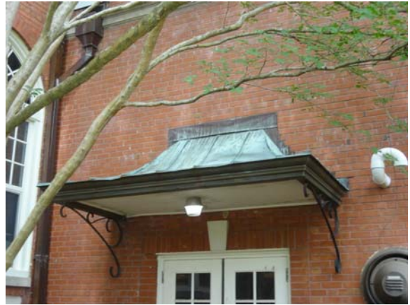
WHIC070a 5/10/2021 One of three copper clad entry canopies South elevation of east wing addition
