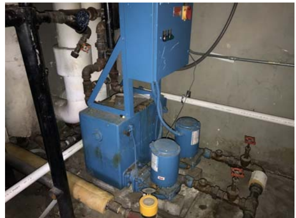
WHIC030e 5/10/2021 Duplex condensate receiver Room 117D
