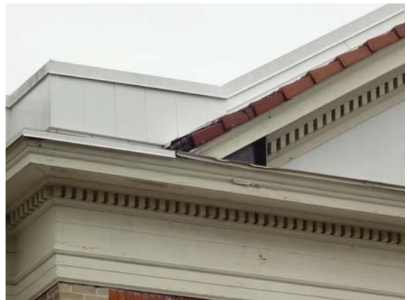
WHIC060a 5/10/2021 Weathering on upper cornice Upper south elevation of original building
