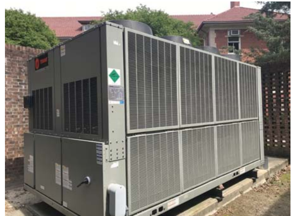
WHIC041e 5/10/2021 Air-cooled packaged chiller Courtyard
