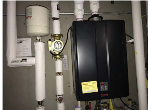
WHIC031e 5/10/2021 Tankless gas-fired water heater with circulation pump Room 117D
