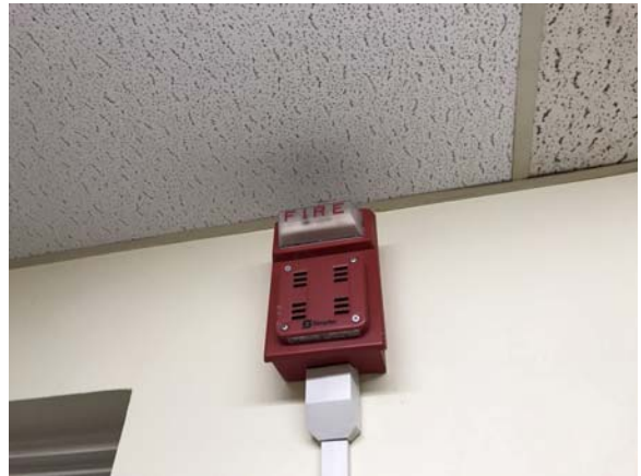
WHIC005e 5/10/2021 Horn with neon strobe Second floor corridor
