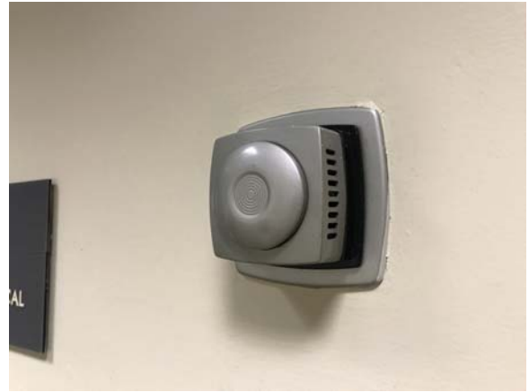
WHIC019e 5/10/2021 Local pneumatic thermostat First floor corridor
