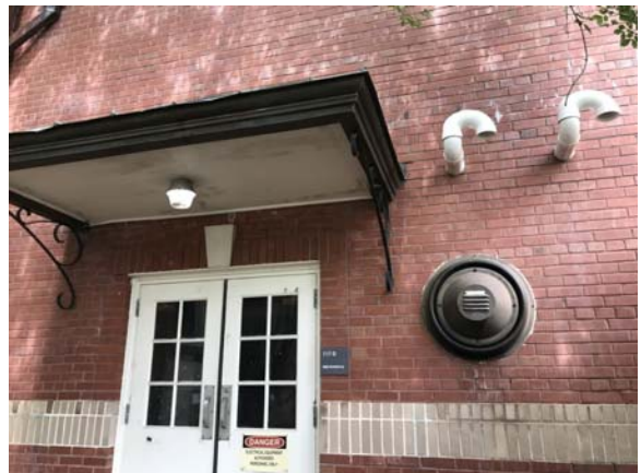
WHIC039e 5/10/2021 Centrifugal exhaust fan Entry
