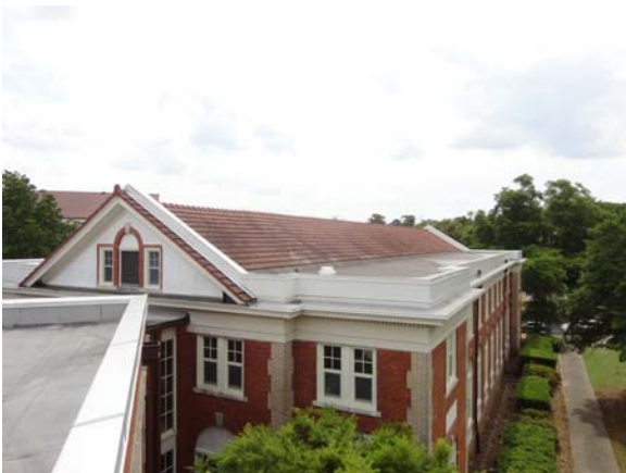
WHIC003a 5/10/2021 Older pitched clay tile roof and newer flat side roof Main roof
