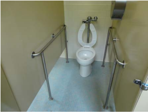
WHIC037a 5/10/2021 Partially accessible toilet stall First floor, men's restroom
