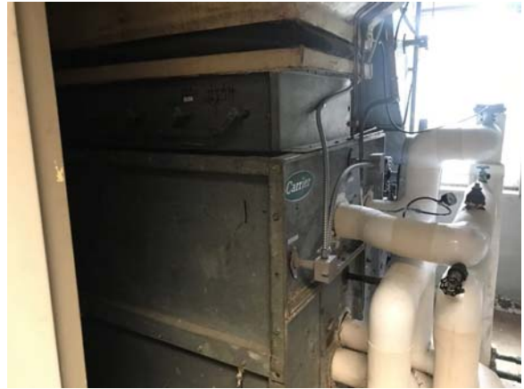
WHIC022e 5/10/2021 Air handling unit AHU-001 Room 108
