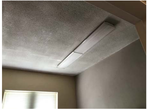
WHIC004e 5/10/2021 Retrofitted T8 troffer lighting fixture Stairwell
