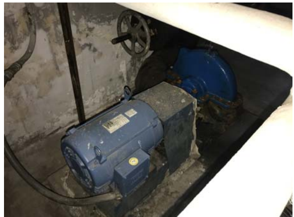
WHIC036e 5/10/2021 Chilled water pump Room 117D
