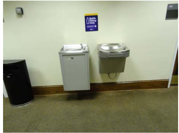
WHIC044a 5/10/2021 Two older water fountains set at same height First floor, original building corridor
