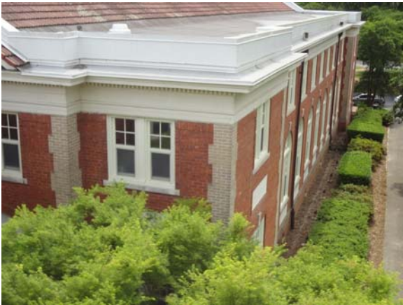
WHIC005a 5/10/2021 Upper wood cornice work and wood trim have peeling paint Upper exterior of main building
