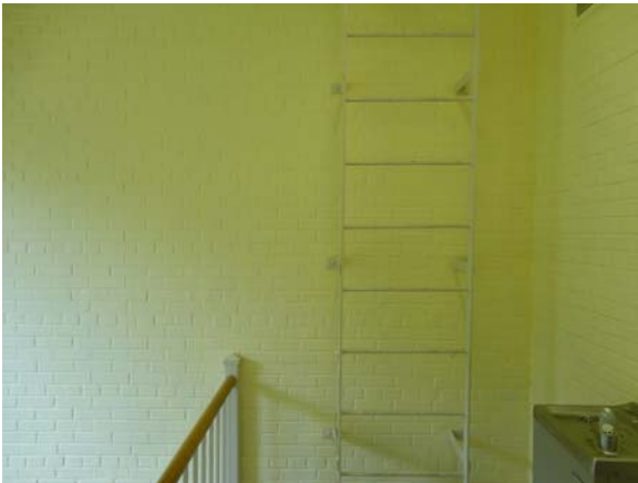
WHIC008a 5/10/2021 No fall protection for ladder at top of stair tower Second floor, annex stair tower
