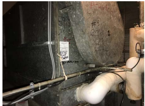
WHIC012e 5/10/2021 Air handling unit AHU-005 Room 214D
