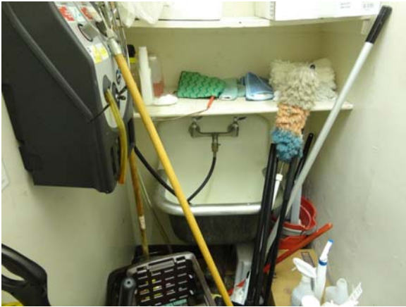
WHIC040a 5/10/2021 Older wall-mounted service sink First floor, janitors closet
