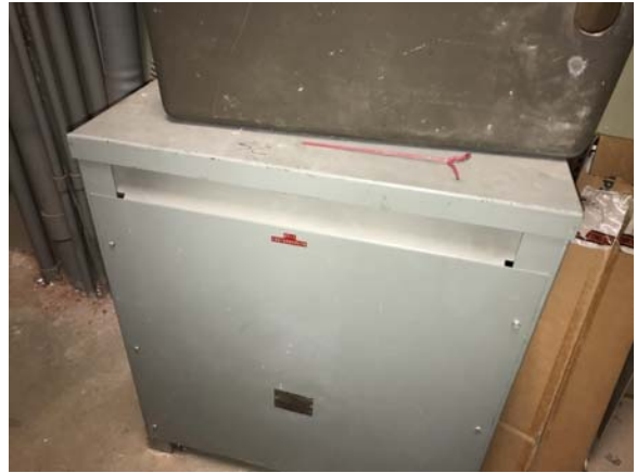
WHIC037e 5/10/2021 Stepdown dry-type transformer Room 119
