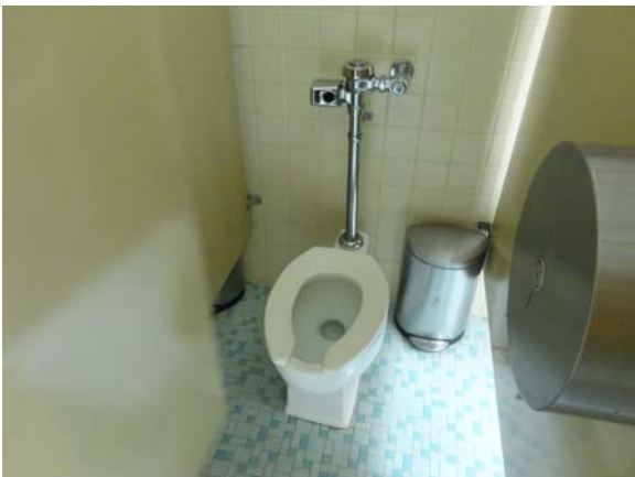
WHIC042a 5/10/2021 Standard tankless water closet First floor, women's restroom
