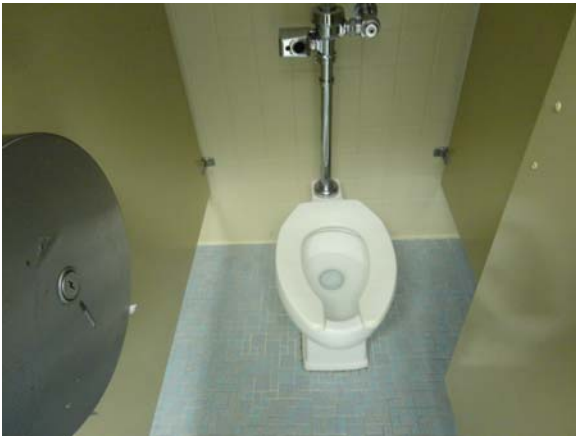
WHIC020a 5/10/2021 Older standard tankless water closet Second floor, men's restroom
