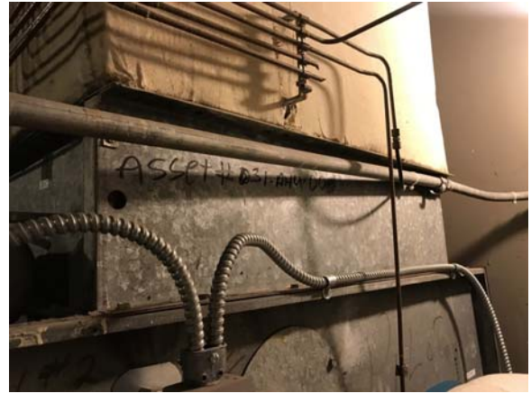
WHIC016e 5/10/2021 Air handling unit AHU-003 Room 118
