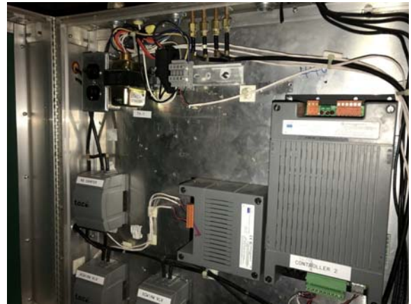
WHIC014e 5/10/2021 Pneumatic HVAC controls Room 214D
