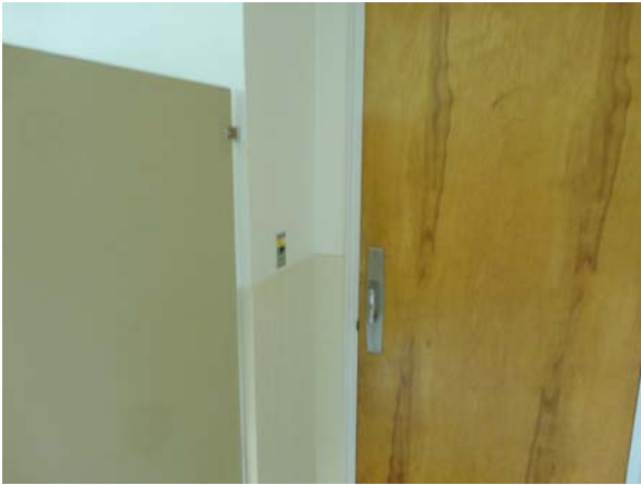
WHIC025a 5/10/2021 Narrow door clearances and restroom entry door Second floor, women's restroom
