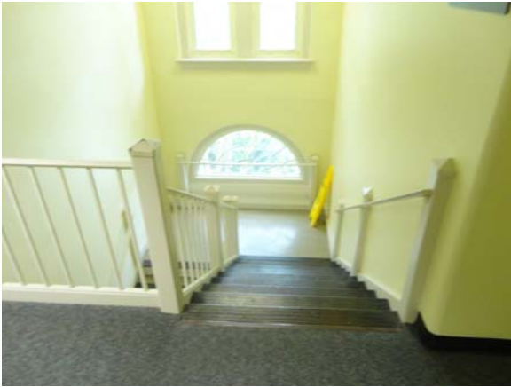
WHIC028a 5/10/2021 Nonaccessible railing detail on stair tower Second floor, original stair tower
