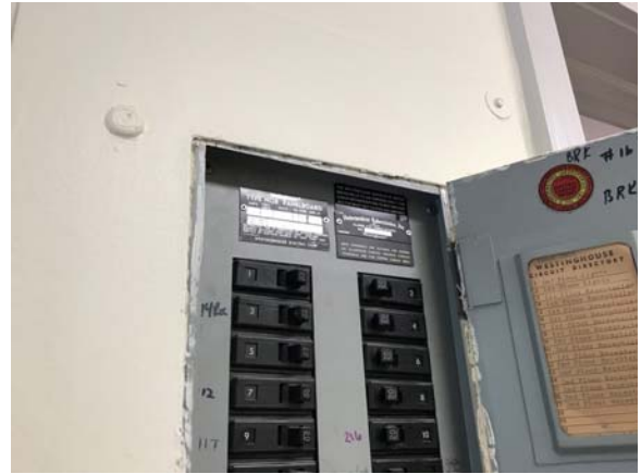
WHIC007e 5/10/2021 Vintage local panelboard Second floor corridor
