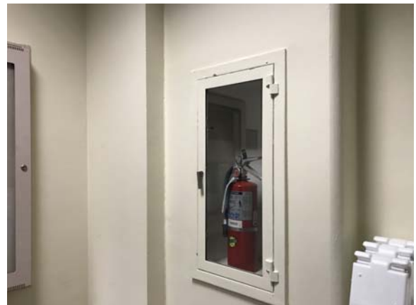
WHIC021e 5/10/2021 Fire extinguisher First floor corridor
