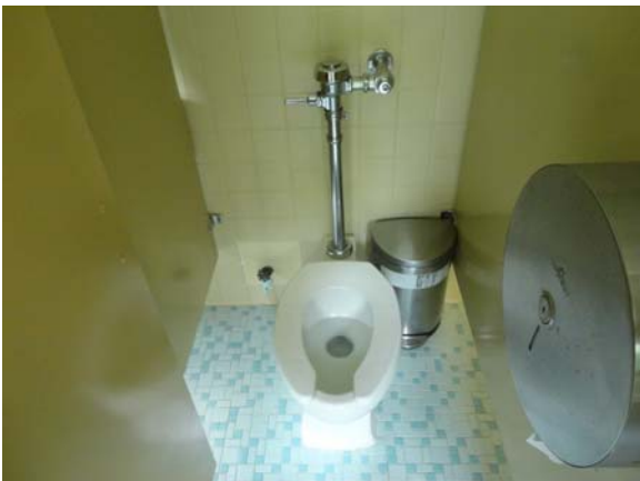
WHIC024a 5/10/2021 Older standard tankless water closet Second floor, women's restroom
