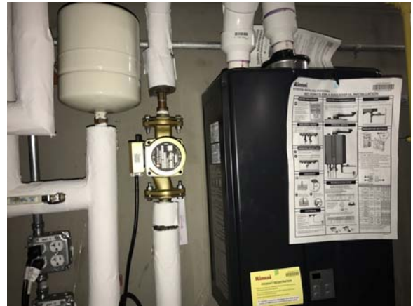
WHIC032e 5/10/2021 Tankless gas-fired water heater with circulation pump Room 117D
