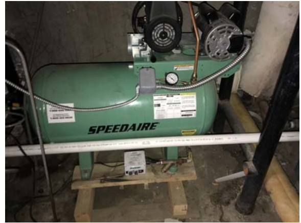
WHIC028e 5/10/2021 Controls air compressor Room 117D
