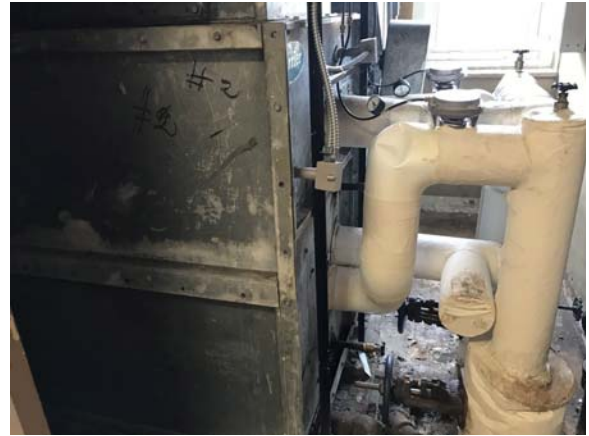
WHIC001e 5/10/2021 Air handling unit AHU-002 Room 227
