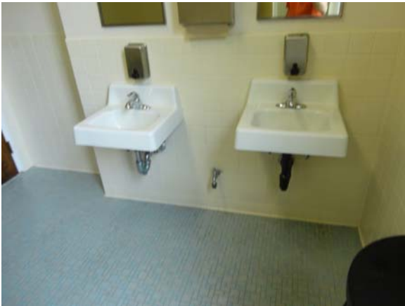
WHIC038a 5/10/2021 Wall-hung lavatories First floor, men's restroom
