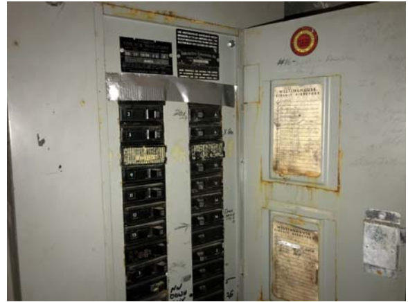
WHIC010e 5/10/2021 Vintage local panelboard Room 214D
