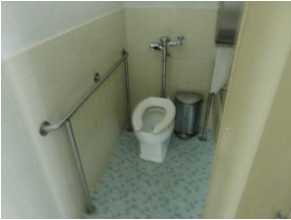
WHIC043a 5/10/2021 Partially accessible toilet stall First floor, women's restroom
