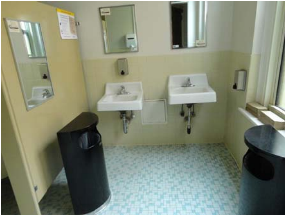
WHIC041a 5/10/2021 Wall-hung lavatories First floor, women's restroom
