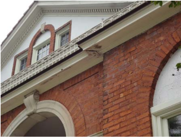
WHIC069a 5/10/2021 Localized dry rot on soffit South elevation
