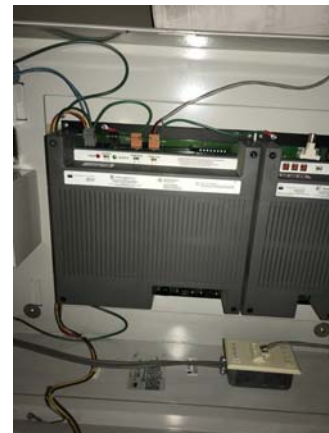
WHIC033e 5/10/2021 DDC HVAC controls Room 117D
