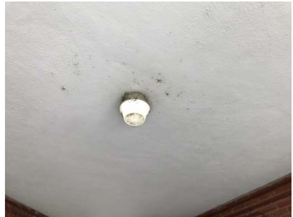
WHIC008e 5/10/2021 Ceiling-mounted HID lighting fixture Second floor, breezeway
