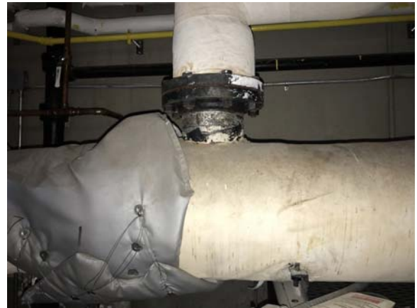
WHIC029e 5/10/2021 Heating hot water shell-and-tube heat exchanger Room 117D
