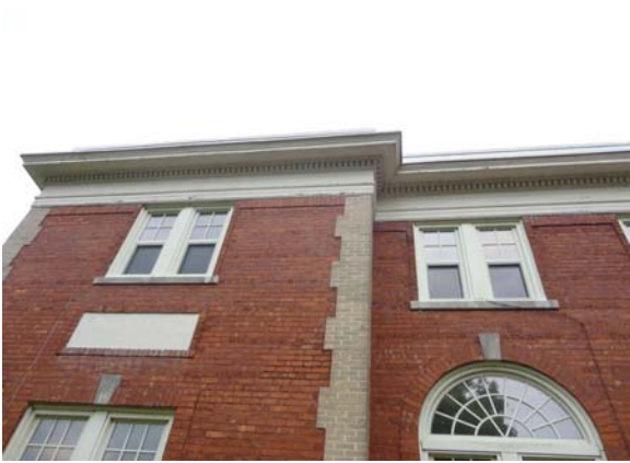
WHIC057a 5/10/2021 Weathered upper wood cornice Upper west elevation of original building
