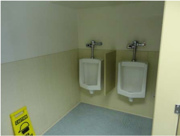
WHIC019a 5/10/2021 Newer wall-hung urinals Second floor, men's restroom
