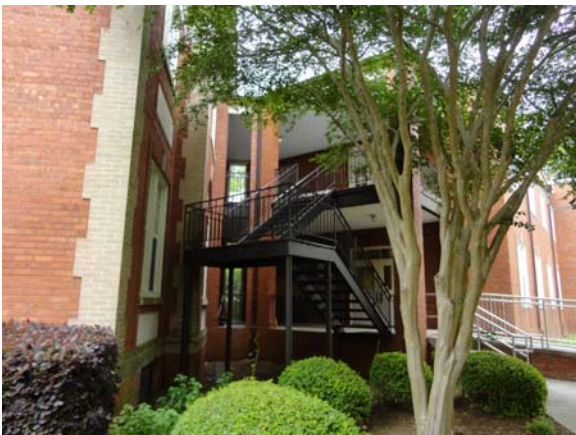
WHIC065a 5/10/2021 Aging exterior metal egress stair with open risers Northeast breezeway
