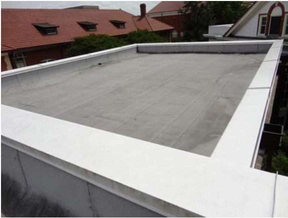
WHIC004a 5/10/2021 Metal cap flashing detail on low parapet wall Annex roof perimeter
