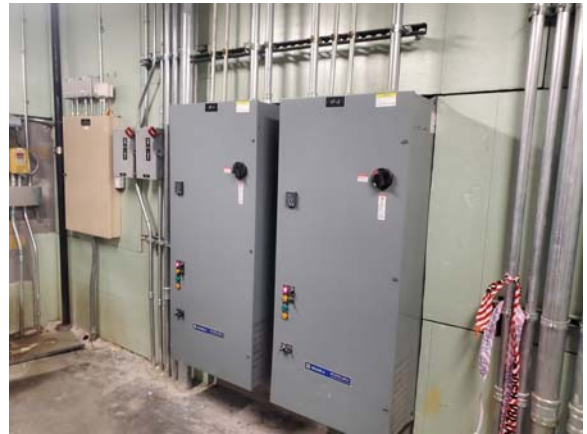
MCCP1044e 4/6/2022 VFDs for towers CT-1 and CT-2 CCP#1 Cooling Tower mezzanine
