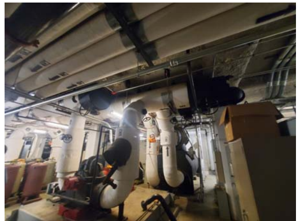
MCCP1024e 4/6/2022 Various distribution piping Science & Tech room C101
