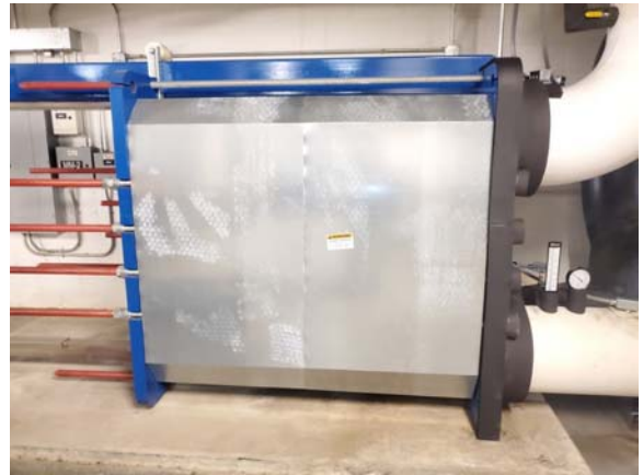
MCCP1008e 4/6/2022 Free cooling plate-and-frame heat exchanger Science & Tech room C101
