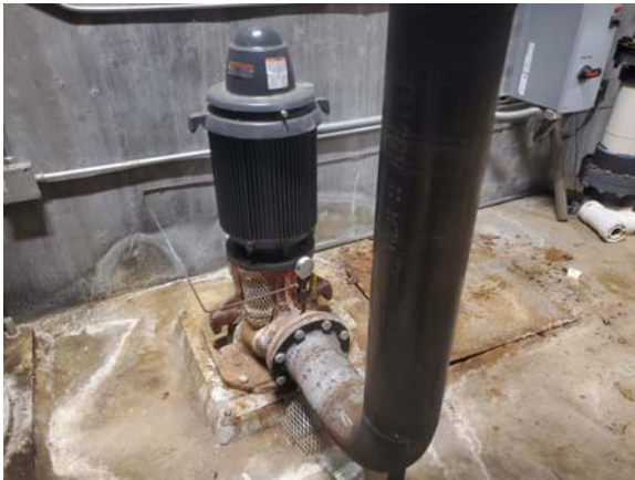
MCCP1037e 4/6/2022 Filter pump CCP#1 Cooling Tower room 100
