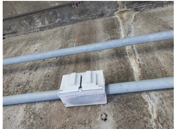
MCCP1058e 4/6/2022 Secondary electrical outlet CCP#1 Cooling Tower roof
