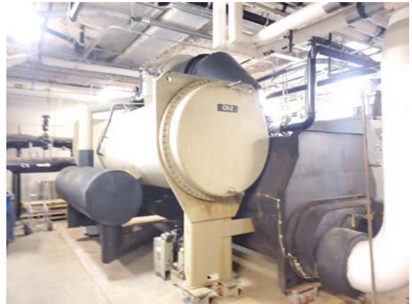
MCCP1010e 4/6/2022 1,470-ton, water-cooled chiller CH-2 Science & Tech room C101
