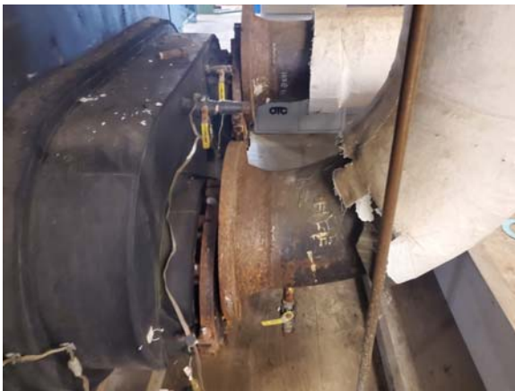
MCCP1023e 4/6/2022 Chiller CH-4 under maintenance Science & Tech room C101
