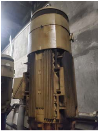
MCCP1031e 4/6/2022 CHP-1 motor assembly CCP#1 Cooling Tower room 100
