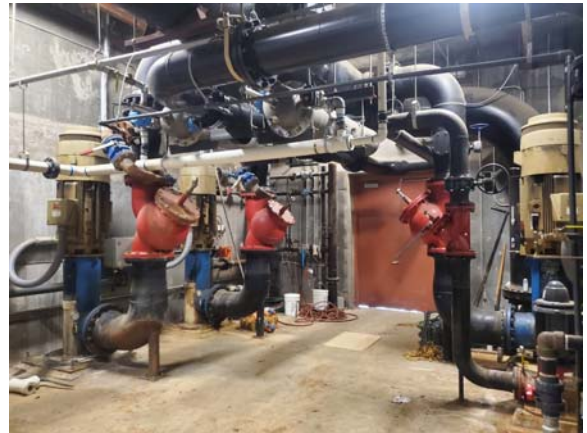
MCCP1040e 4/6/2022 Overview of condenser water pump room CCP#1 Cooling Tower room 100
