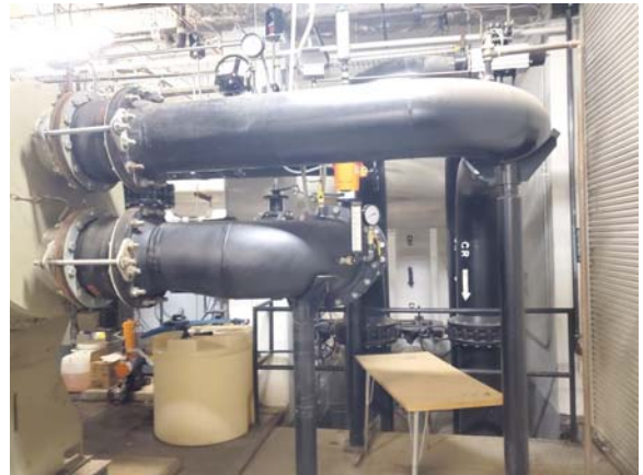
MCCP1002e 4/6/2022 Condenser water pipe and valves Science & Tech room C101
