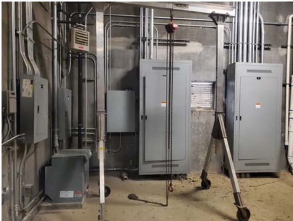
MCCP1039e 4/6/2022 Various secondary electric equipment CCP#1 Cooling Tower room 100
