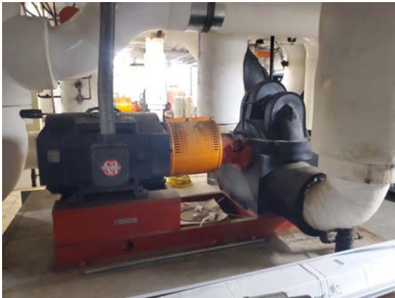
MCCP1007e 4/6/2022 Chilled water pump CHP-1 Science & Tech room C101
