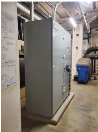
MCCP1017e 4/6/2022 Chiller CH-1 motor starter Science & Tech room C101
