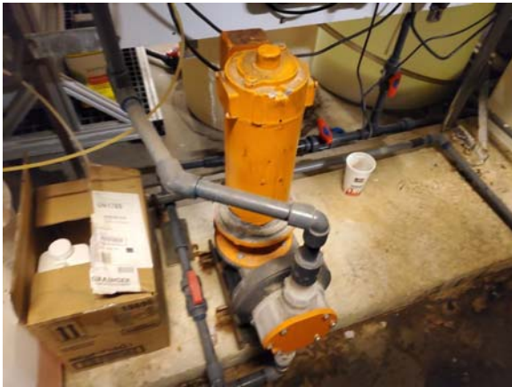
MCCP1001e 4/6/2022 Water treatment chemical feeder pump Science & Tech room C101
