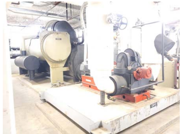
MCCP1012e 4/6/2022 Chiller CH-3 and pump CHP-3 Science & Tech room C101
