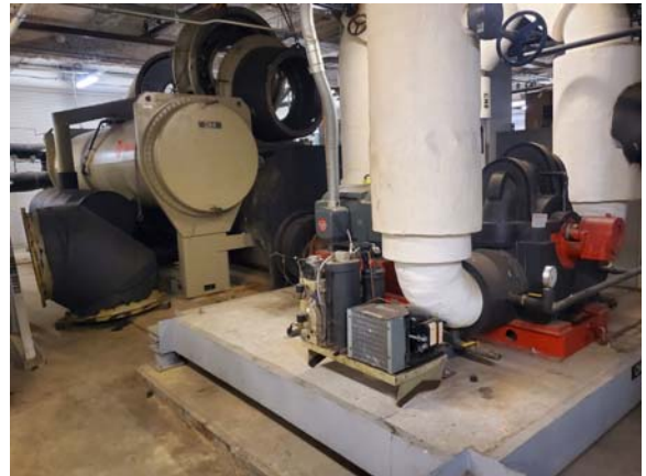
MCCP1022e 4/6/2022 Chiller CH-4 and pump CHP-4 Science & Tech room C101
