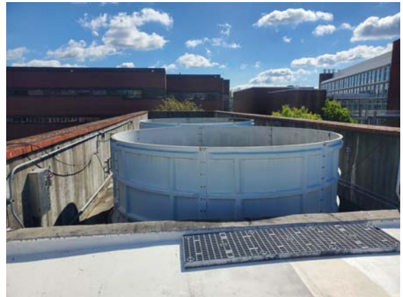
MCCP1052e 4/6/2022 Overview of tower fan assemblies CT-5 to CT-6 CCP#1 Cooling Tower roof
