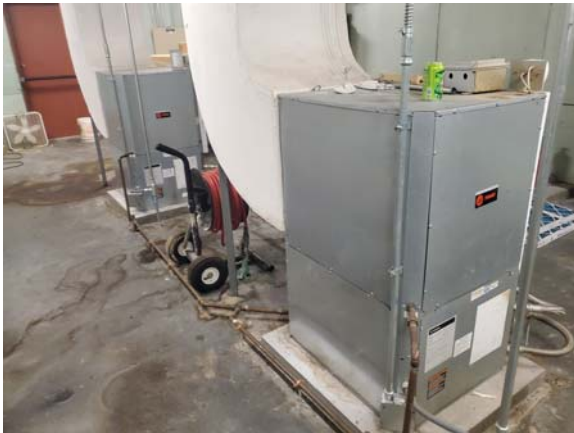
MCCP1045e 4/6/2022 Water source heat pumps AHU-1 and AHU-2 CCP#1 Cooling Tower mezzanine
