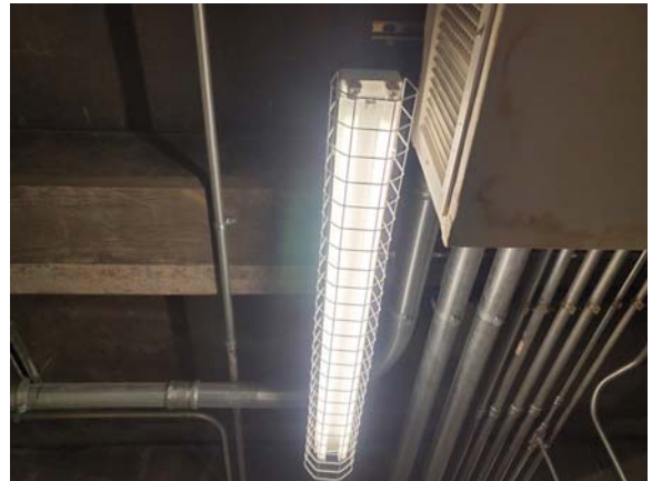
MCCP1064e 4/6/2022 Surface-mounted, interior lighting with T8 lamps CCP#1 Cooling Tower room 100
