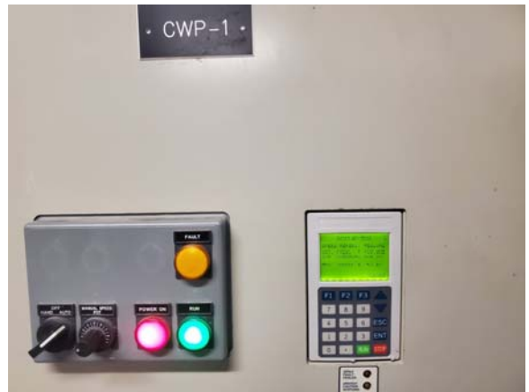
MCCP1048e 4/6/2022 Deficient display for VFD CWP-1 CCP#1 Cooling Tower mezzanine
