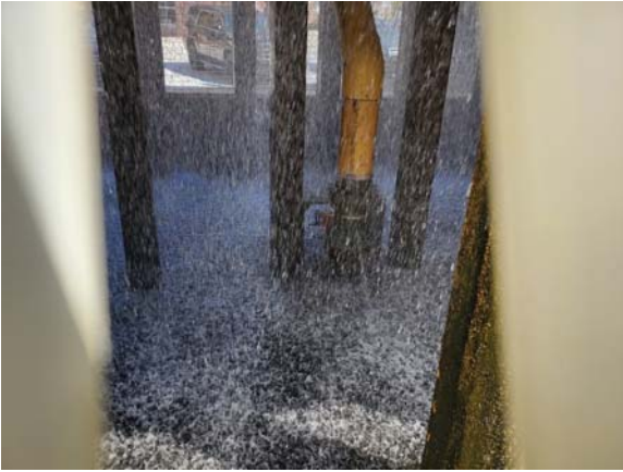
MCCP1067e 4/6/2022 Leaking inlet water pipe and union CCP#1 Cooling Tower basin
