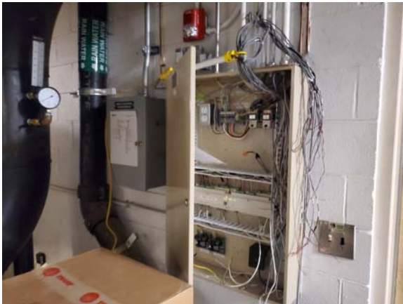
MCCP1015e 4/6/2022 Chiller Water Plant energy panel Science & Tech room C101
