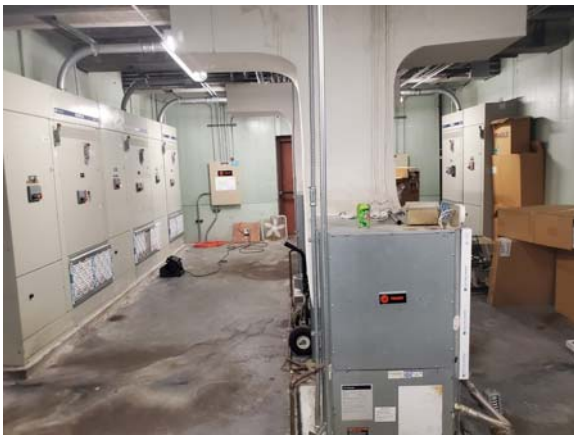
MCCP1041e 4/6/2022 Overview of drive room CCP#1 Cooling Tower mezzanine
