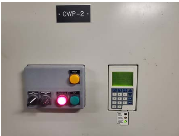
MCCP1047e 4/6/2022 Deficient display for VFD CWP-2 CCP#1 Cooling Tower mezzanine
