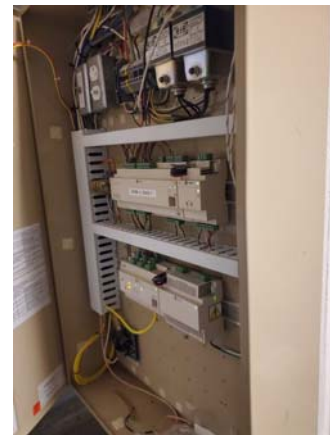
MCCP1018e 4/6/2022 Chiller 1 control panel Science & Tech room C101
