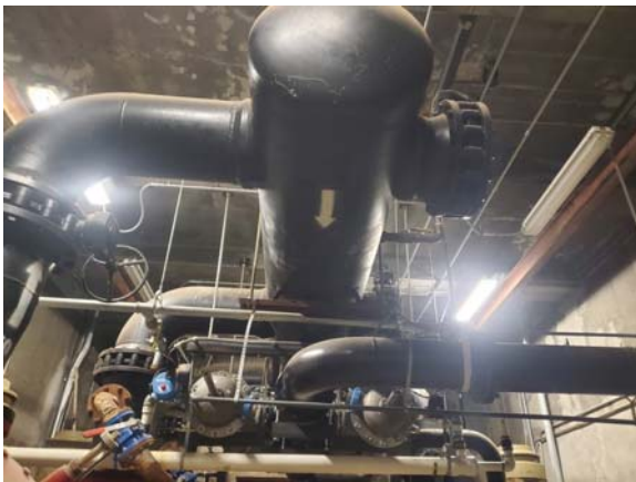
MCCP1035e 4/6/2022 Condenser water combined header and filtration CCP#1 Cooling Tower room 100
