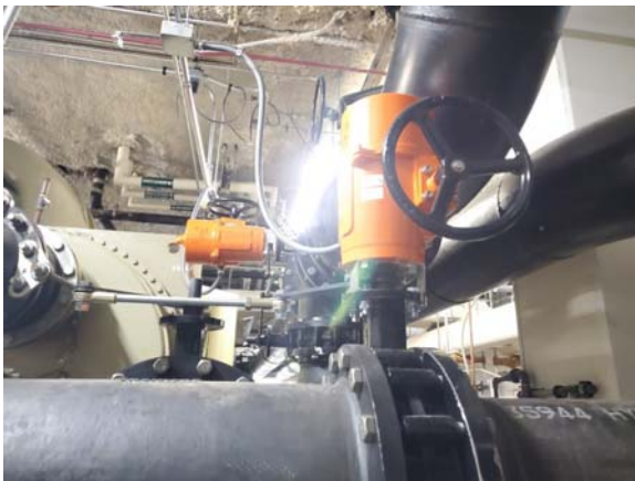
MCCP1005e 4/6/2022 Electronically operated isolation valves Science & Tech room C101
