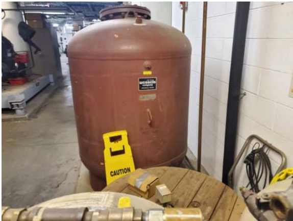
MCCP1021e 4/6/2022 422-gallon chilled water expansion tank Science & Tech room C101
