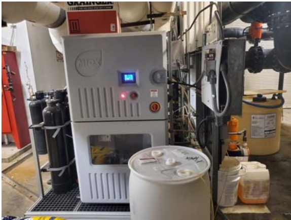
MCCP1013e 4/6/2022 MIOX water treatment system Science & Tech room C101
