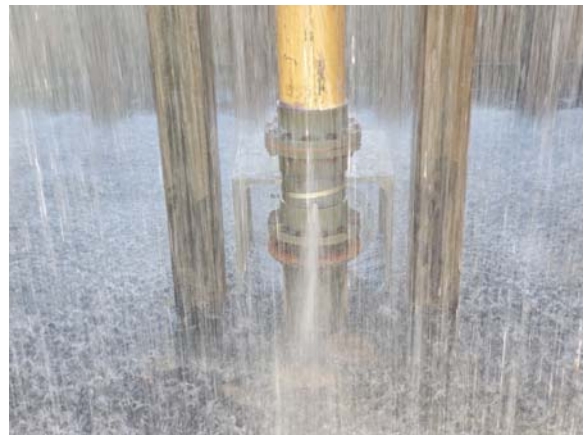
MCCP1066e 4/6/2022 Leaking inlet water pipe and union CCP#1 Cooling Tower basin
