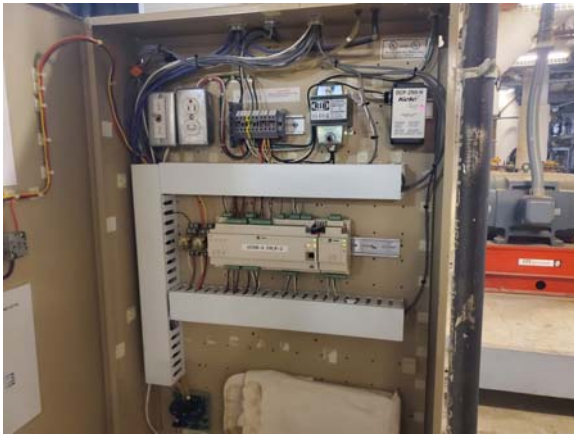
MCCP1019e 4/6/2022 Chiller 2 control panel Science & Tech room C101
