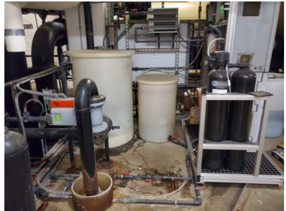
MCCP1014e 4/6/2022 Water softening and treatment equipment Science & Tech room C101
