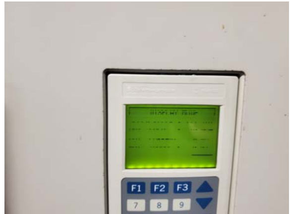
MCCP1046e 4/6/2022 Deficient display for VFD CWP-3 CCP#1 Cooling Tower mezzanine
