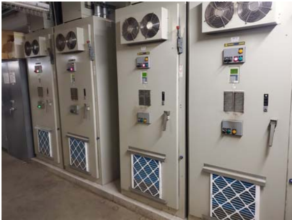
MCCP1025e 4/6/2022 Aged variable speed drives for the chilled water pumps Science & Tech room C101
