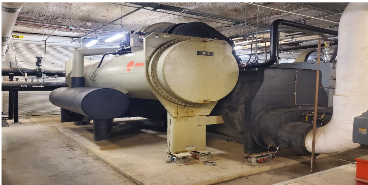
Image 1: 1,470 water-cooled chiller CH-3
