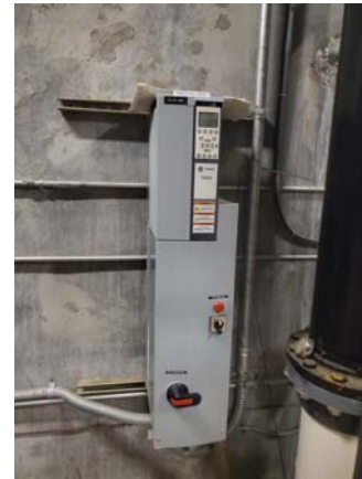
MCCP1038e 4/6/2022 Filter pump variable speed drive CCP#1 Cooling Tower room 100
