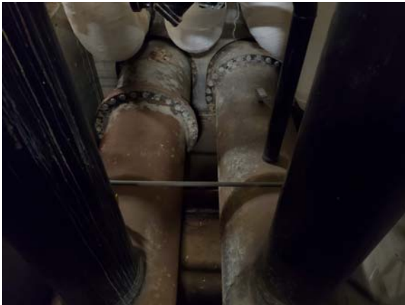
MCCP1003e 4/6/2022 Condenser water pipe Science & Tech room C101
