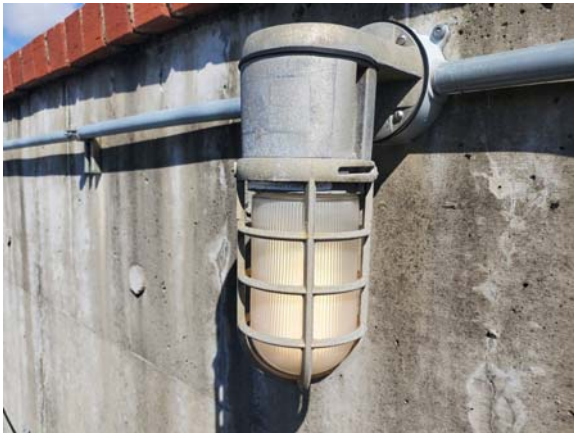
MCCP1057e 4/6/2022 Surface-mounted exterior lighting CCP#1 Cooling Tower roof
