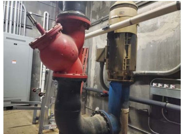
MCCP1034e 4/6/2022 Condenser water pump CHP-3 CCP#1 Cooling Tower room 100
