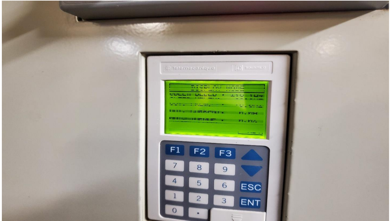
Image 3: Deficient variable speed drive display
