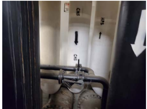
MCCP1004e 4/6/2022 Chilled water supply and return pipe to campus Science & Tech room C101
