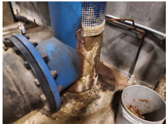
MCCP1030e 4/6/2022 Condenser water pump 1 with minor scale and corrosion CCP#1 Cooling Tower room 100
