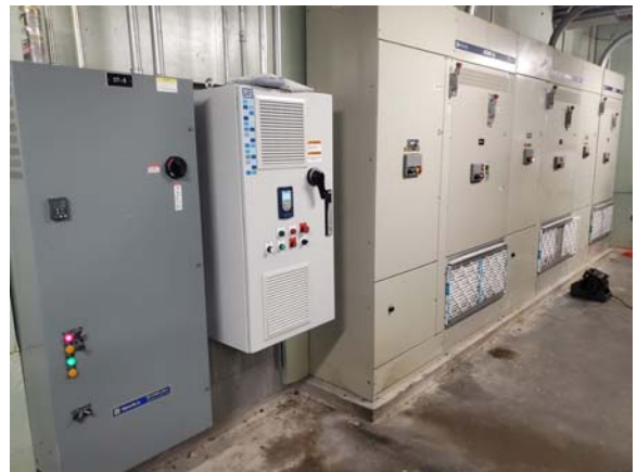
MCCP1042e 4/6/2022 VFDs for pumps CWP-1 to CWP-3 and towers CT-3 and CT-4 CCP#1 Cooling Tower mezzanine
