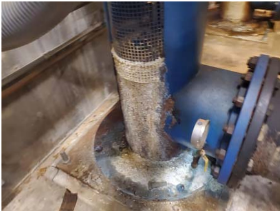
MCCP1033e 4/6/2022 Condenser water pump 2 with minor scale and corrosion CCP#1 Cooling Tower room 100
