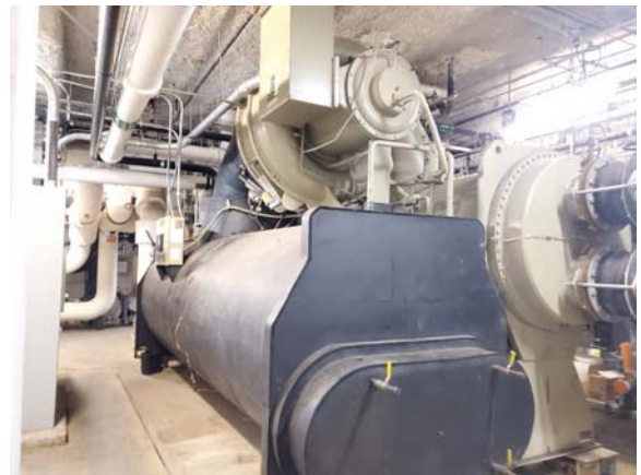
MCCP1006e 4/6/2022 1,470-ton, water-cooled chiller CH-1 Science & Tech room C101
