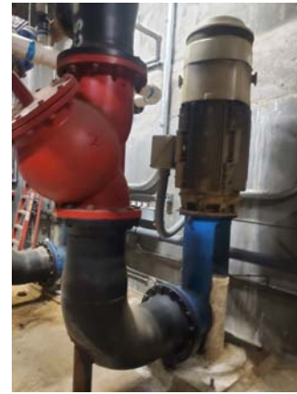
MCCP1032e 4/6/2022 Condenser water pump CHP-2 CCP#1 Cooling Tower room 100
