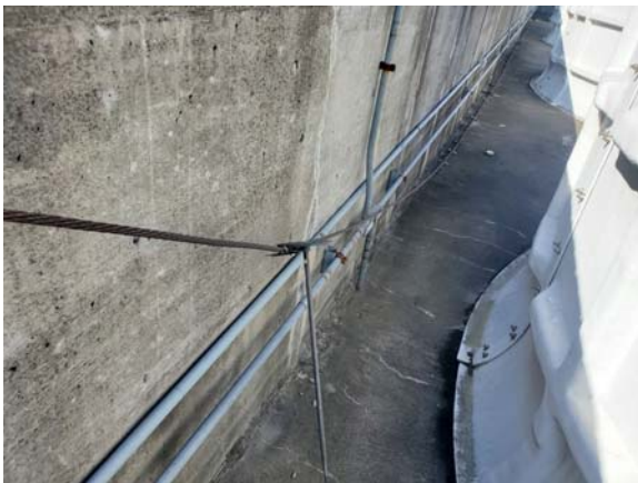
MCCP1059e 4/6/2022 Damaged lightning protection CCP#1 Cooling Tower roof
