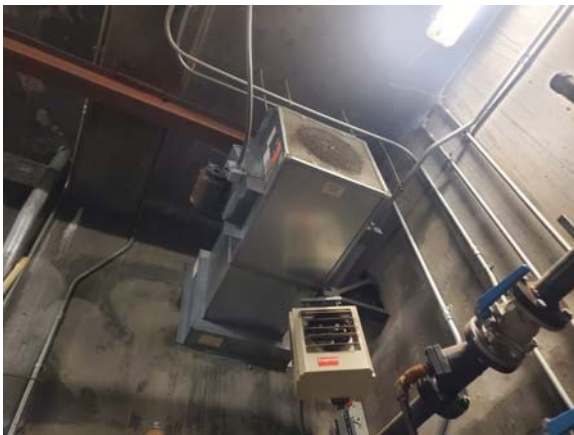
MCCP1029e 4/6/2022 Fan and electric unit heater CCP#1 Cooling Tower room 100
