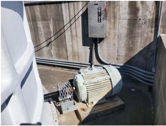
MCCP1055e 4/6/2022 Cooling tower CT-1 fan motor CCP#1 Cooling Tower roof
