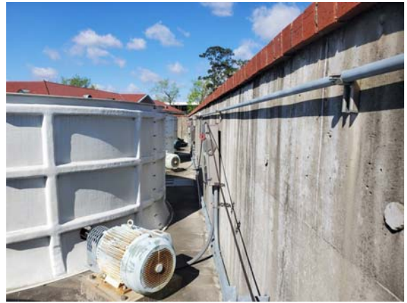
MCCP1056e 4/6/2022 Damaged lightning protection CCP#1 Cooling Tower roof
