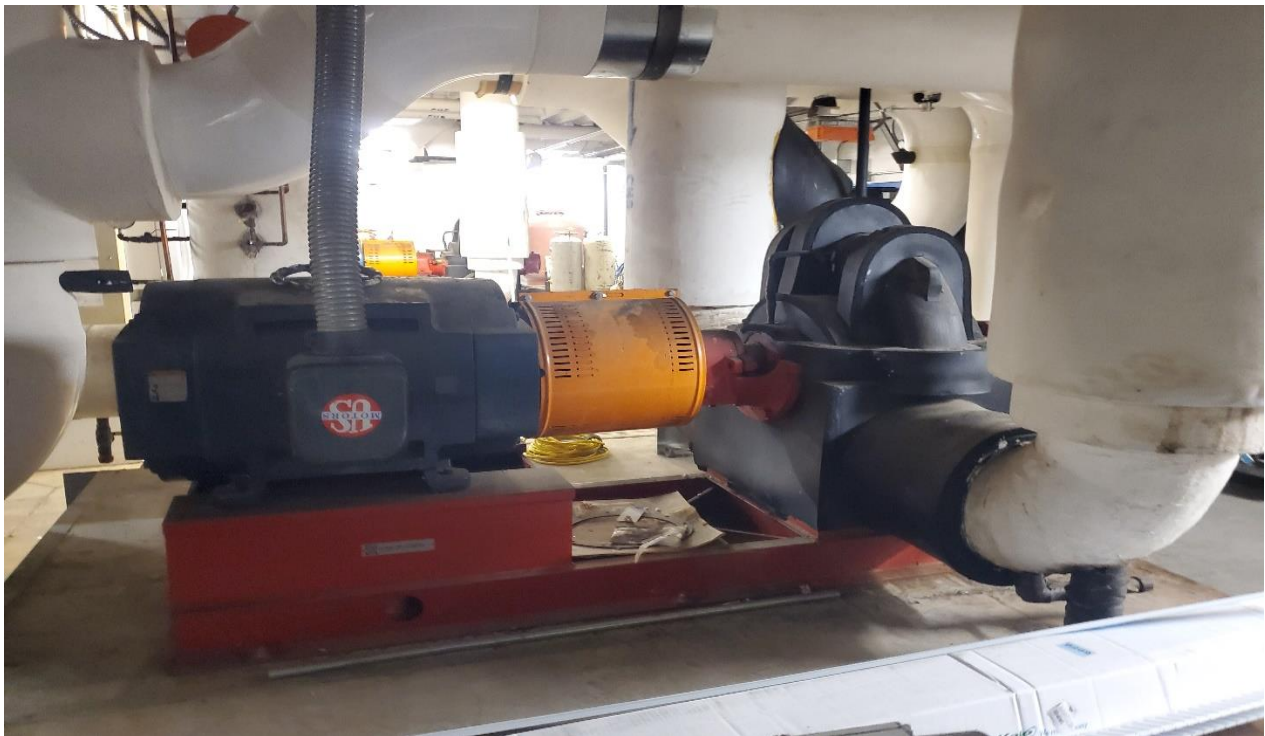
Image 2: Chilled water pump CHP-1
