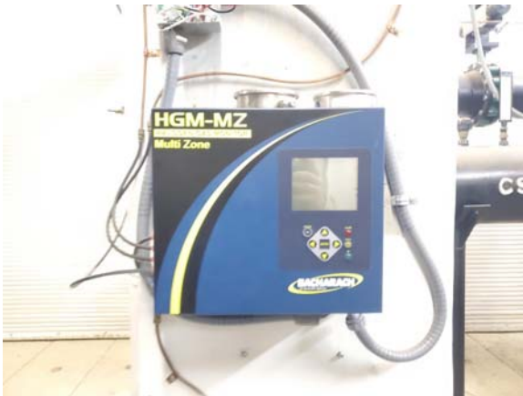
MCCP1011e 4/6/2022 Refrigerant monitoring system Science & Tech room C101
