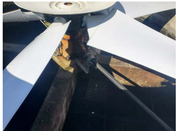
MCCP1054e 4/6/2022 Cooling tower CT-1 fan gear box CCP#1 Cooling Tower roof
