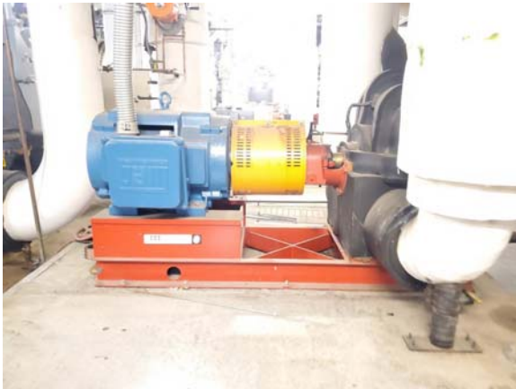
MCCP1009e 4/6/2022 Chilled water pump CHP-2 Science & Tech room C101
