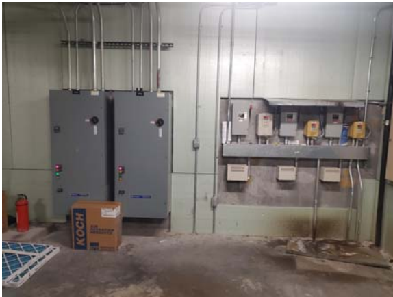
MCCP1043e 4/6/2022 VFDs for towers CT-5 and CT-6 and well pumps CCP#1 Cooling Tower mezzanine
