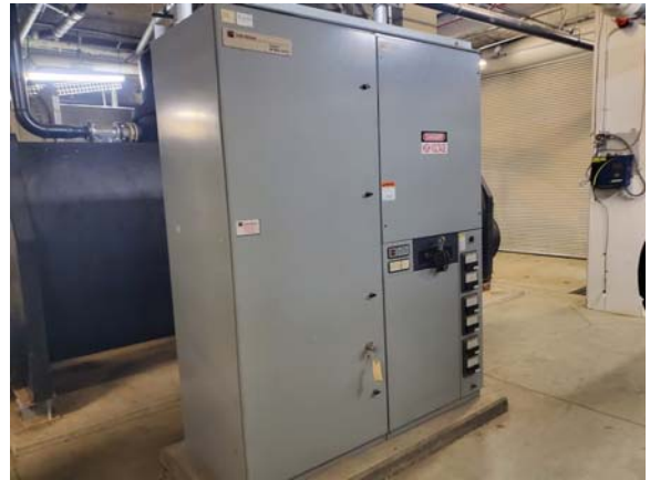
MCCP1020e 4/6/2022 Chiller CH-2 motor starter Science & Tech room C101
