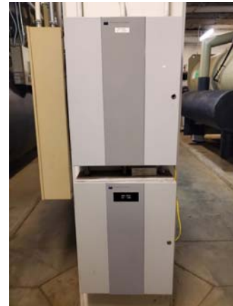
MCCP1016e 4/6/2022 Chilled Water Plant controls Science & Tech room C101
