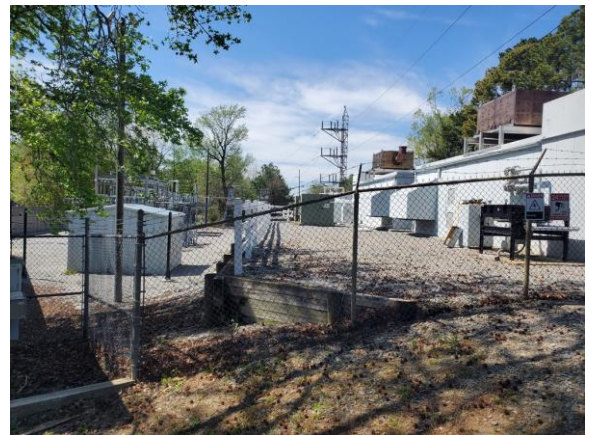
MELEC006e 3/24/2022 Overview of GUCO substation Ficklen Drive
