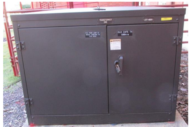
MELEC024e 3/24/2022 Old Cafeteria 500 kVA transformer Old Cafeteria, exterior
