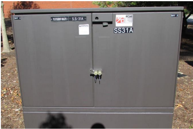
MELEC015e 3/24/2022 Live front sectionalizing switch SS-31A Joyner Clock Tower, exterior
