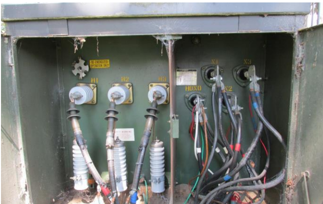
MELECO11e 3/24/2022 Erwin transformer Erwin, exterior
