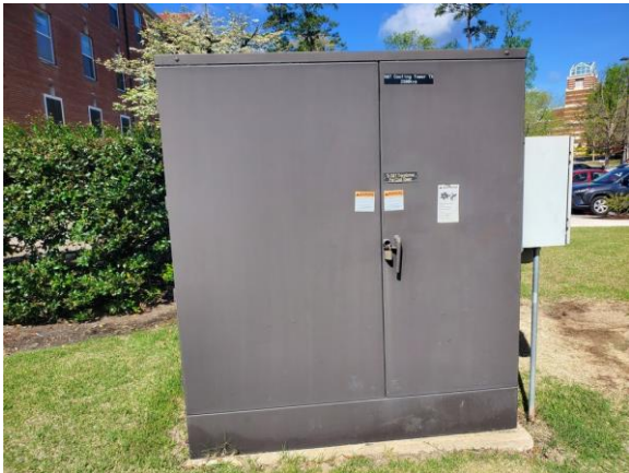
MELEC003e 3/24/2022 2,500 kVA oil-filled transformer S&T Cooling Tower, exterior
