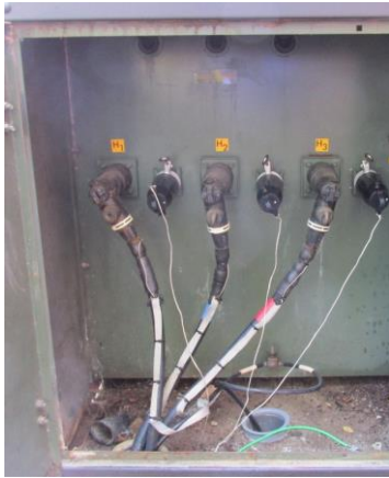
MELEC025e 3/24/2022 Old Cafeteria 500 kVA transformer interior Old Cafeteria, exterior
