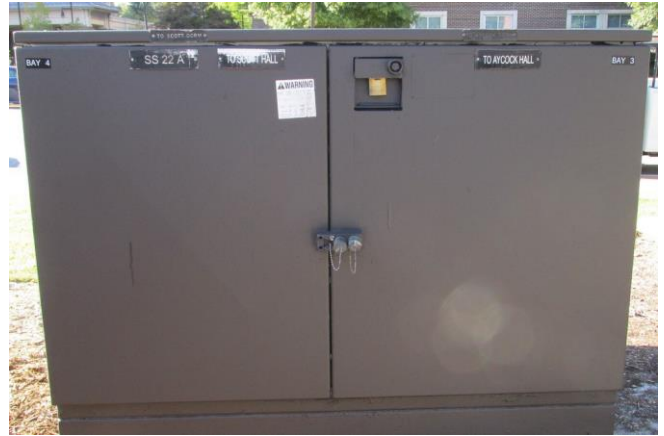
MELEC020e 3/24/2022 Live front sectionalizing switch SS-22A Scott, exterior
