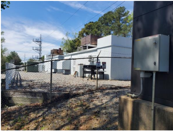
MELECO07e 3/24/2022 Overview of GUCO substation Ficklen Drive
