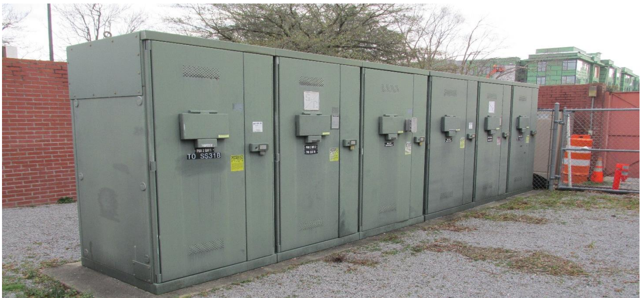
Image 1: Main electrical system Switchgear-3
