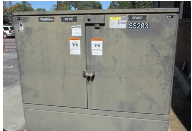
MELECO12e 3/24/2022 Live front sectionalizing switch SS-203 Jenkins Art, exterior
