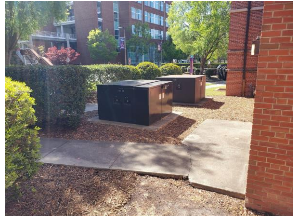
MELEC004e 3/24/2022 Dead front sectionalizing switches SS-30 and SS-38 S&T Cooling Tower, exterior
