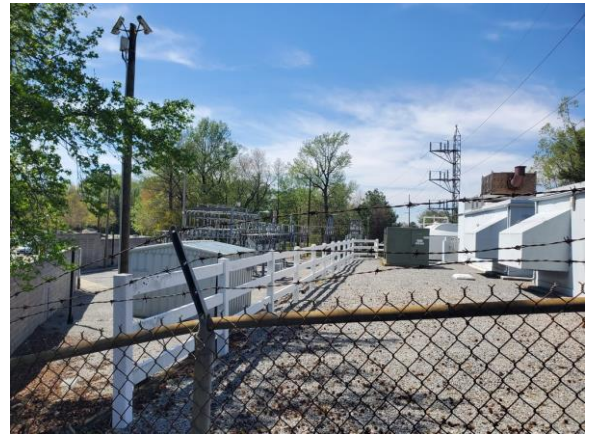
MELECO08e 3/24/2022 Overview of GUCO substation Ficklen Drive
