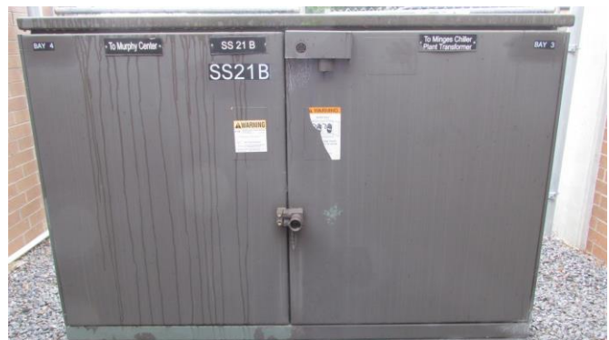
MELEC018e 3/24/2022 Live front sectionalizing switch SS-21B Minges, exterior
