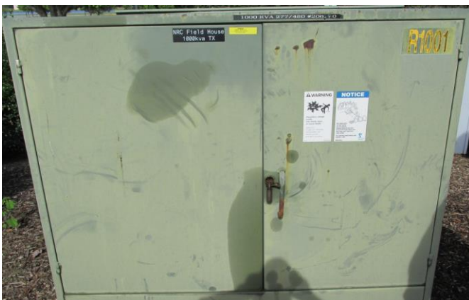
MELEC023e 3/24/2022 NRC Fieldhouse 1000 kVA transformer NRC Fieldhouse, exterior
