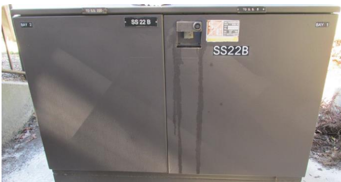
MELEC017e 3/24/2022 Live front sectionalizing switch SS-22B Jones, exterior
