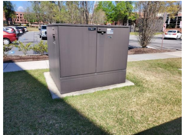
MELEC002e 3/24/2022 Live front sectionalizing switch SS-9 S&T Cooling Tower, exterior
