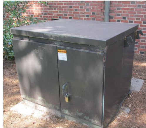
MELECO10e 3/24/2022 Erwin transformer Erwin, exterior
