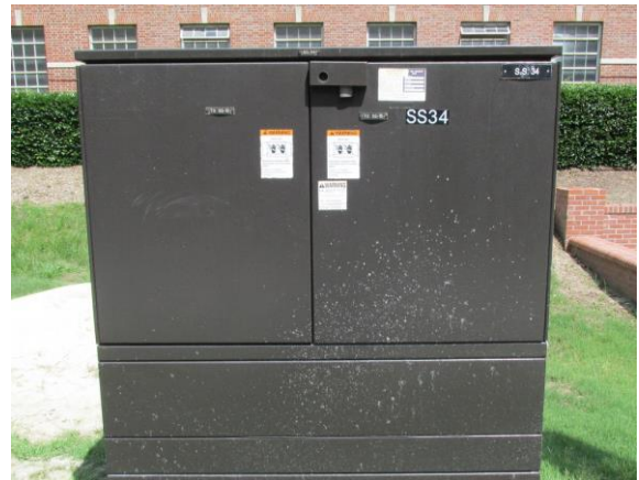
MELEC014e 3/24/2022 Live front sectionalizing switch SS-34 Christenbury, exterior
