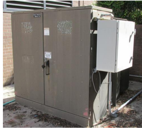
MELEC028e 3/24/2022 Ward 750 kVA transformer Ward, exterior
