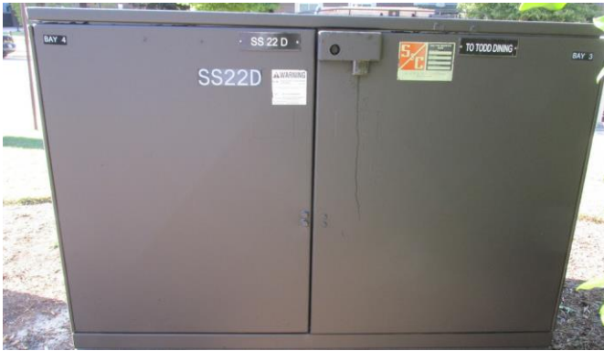
MELEC021e 3/24/2022 Live front sectionalizing switch SS-22D Scott, exterior
