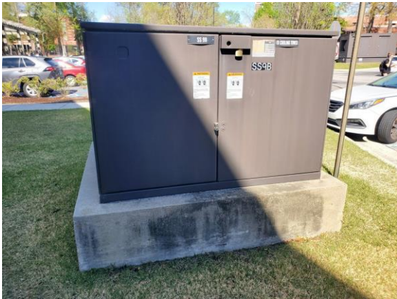
MELEC001e 3/24/2022 Live front sectionalizing switch SS-9B S&T Cooling Tower, exterior
