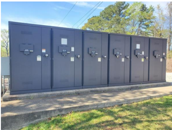
MELEC005e 3/24/2022 Switchgear-1, Pods 1 through 6 Ficklen Drive
