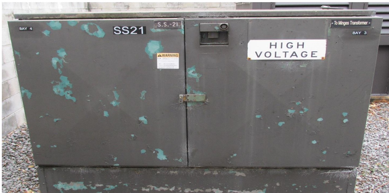
Image 2: Live-front sectionalizing switch SS-21
