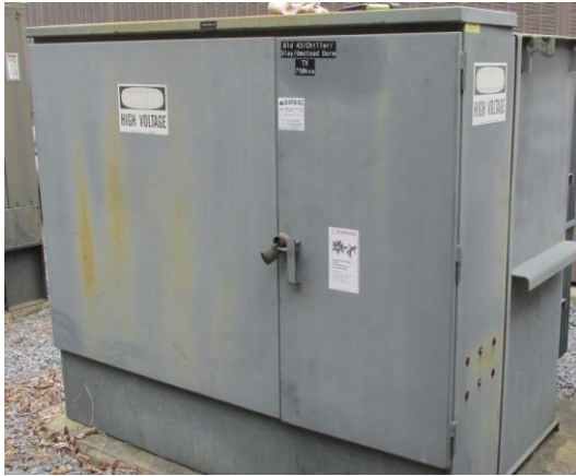
MELEC027e 3/24/2022 B43, Slay, Umstead 750 kVA transformer Umstead, exterior service yard
