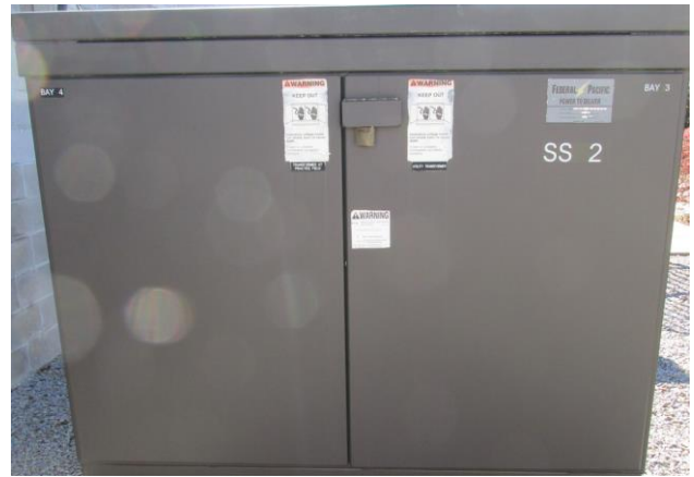
MELEC016e 3/24/2022 Live front sectionalizing switch SS-2 THSC, exterior
