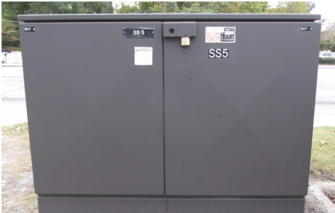
MELEC013e 3/24/2022 Live front sectionalizing switch SS-5 Fletcher Music, exterior
