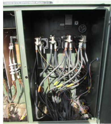
MELEC022e 3/24/2022 NRC Fieldhouse ,1000 kVA transformer interior NRC Fieldhouse, exterior
