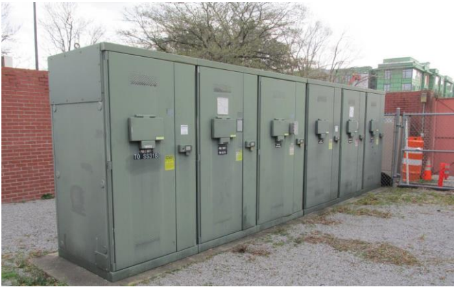
MELECO09e 3/24/2022 Switchgear-3, Pods 1 through 6 Library Drive
