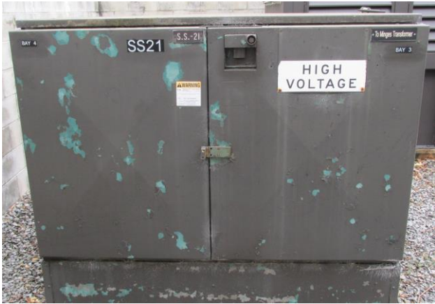
MELEC019e 3/24/2022 Live front sectionalizing switch SS-21 Minges, exterior
