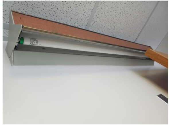
059004e 1/11/2023 Surface-mounted light fixture with T12 fluorescent lamp Waiting room
