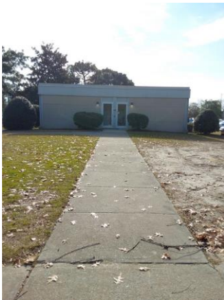
059024a 1/11/2023 Concrete panel facade and exterior glass and aluminum door North elevation
