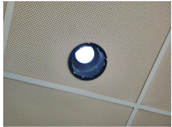
059024e 1/11/2023 Aged recessed light fixture Exterior
