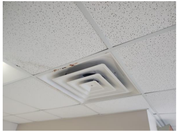
059003e 1/11/2023 HVAC distribution supply/return vent Waiting room
