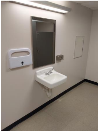
059011a 1/11/2023 Wall-mounted lavatory Men's restroom 113
