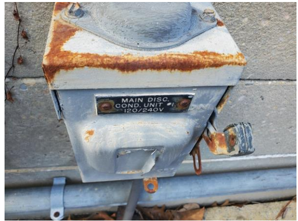
059021e 1/11/2023 Corroded disconnect housing Exterior
