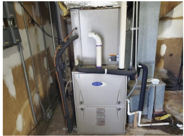
059015e 1/11/2023 Furnace and evaporator coil system #4 Mechanical room 116
