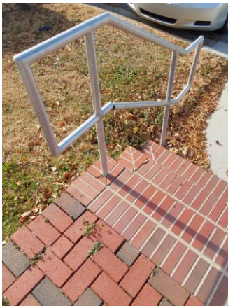
059021a 1/11/2023 Broken exterior entrance stair railing West site
