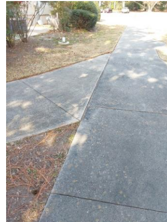
059028a 1/11/2023 Curb bump safety hazard East site
