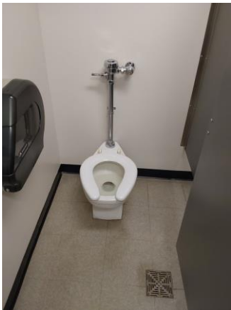
059015a 1/11/2023 Tankless toilet Women's restroom 114
