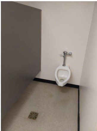
059012a 1/11/2023 Wall-mounted urinal Men's restroom 113
