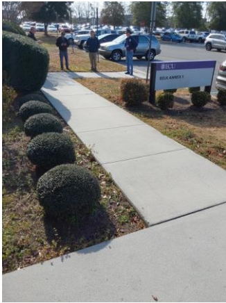
059022a 1/11/2023 Wheelchair ramp without handrail West site
