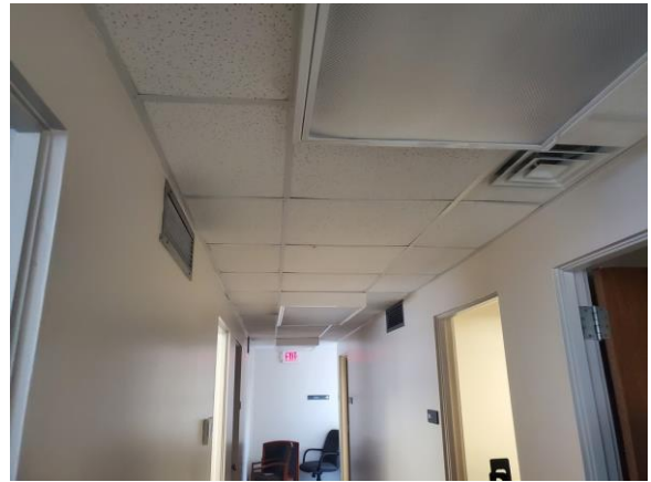
059005e 1/11/2023 Aged, surface-mounted light fixtures Corridor
