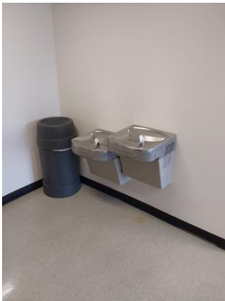
059003a 1/11/2023 Dual-height water fountains Waiting room
