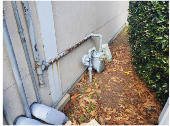
059013e 1/11/2023 Natural gas meter and regulating valve Exterior
