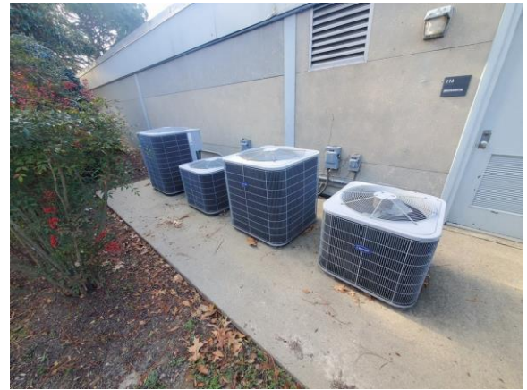
059020e 1/11/2023 Air-cooled condensers Exterior
