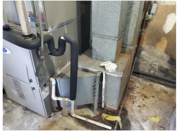
059016e 1/11/2023 Corroded metal ductwork Mechanical room 116
