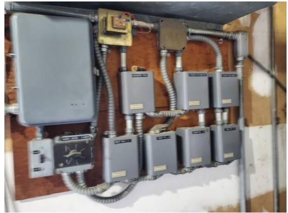
059014e 1/11/2023 Aged electromechanical HVAC equipment starters Mechanical room 116
