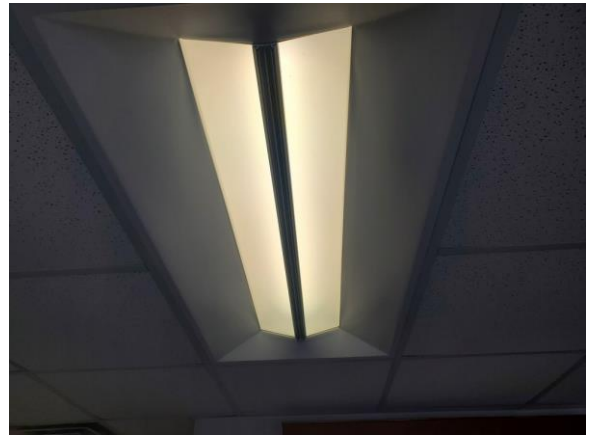
059002e 1/11/2023 2x4 recessed lighting with LED retrofit Waiting room
