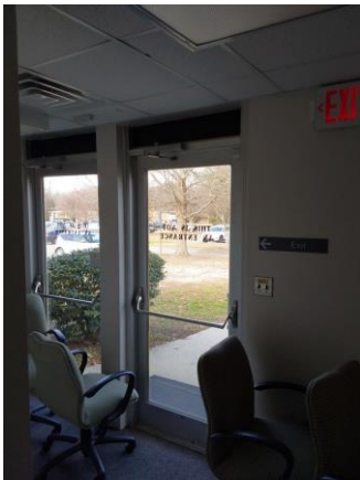
059009a 1/11/2023 Exit doors with old style panic hardware Corridor
