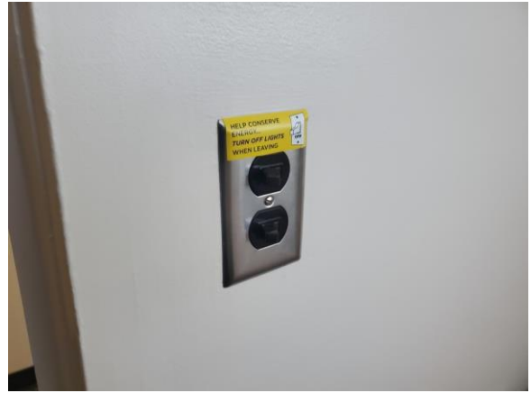
059007e 1/11/2023 Typical secondary electric power outlet Office 101
