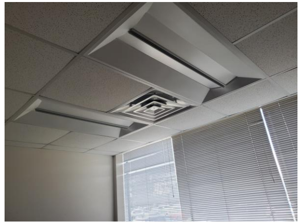
059006e 1/11/2023 2x4 recessed lighting with LED retrofit Office 101
