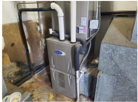
059018e 1/11/2023 Furnace and evaporator coil system #3 Mechanical room 116
