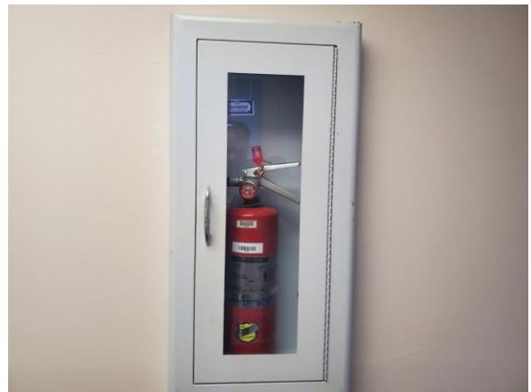
059008e 1/11/2023 Dry chemical fire extinguisher Corridor
