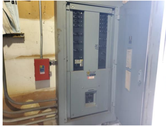
059019e 1/11/2023 120/240 volt, 350 amp main electrical panel Mechanical room 116
