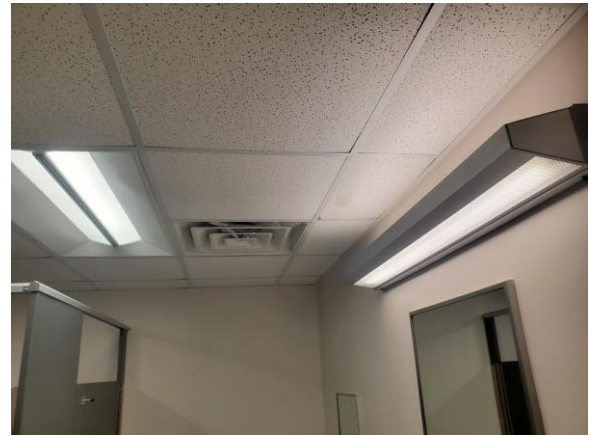
059011e 1/11/2023 Interior lighting and HVAC diffuser Women's restroom 114
