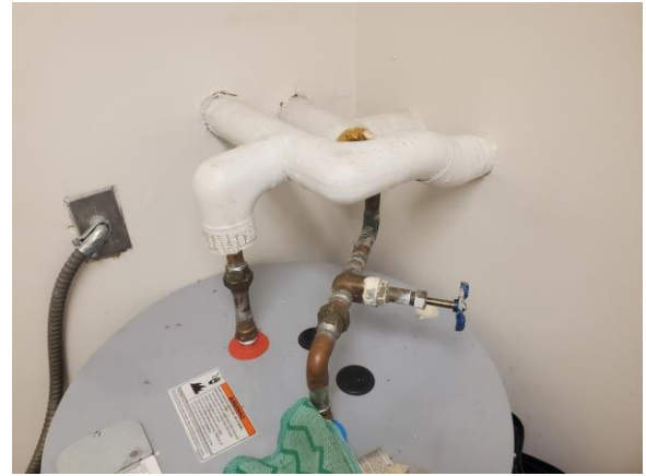
059010e 1/11/2023 Copper supply piping Custodial room 115
