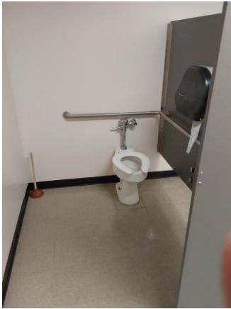
059013a 1/11/2023 Tankless toilet Men's restroom 113
