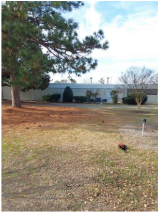
059025a 1/11/2023 Concrete panel facade, glass and aluminum exterior door, and louver East elevation
