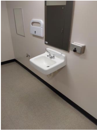
059016a 1/11/2023 Wall-mounted lavatory Women's restroom 114
