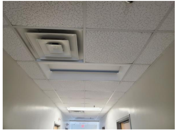
013019e 1/11/2023 2x4 recessed lighting with LED retrofit Corridor 3004
