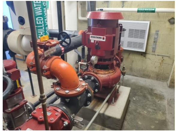
013062e 1/11/2023 Main fire pump Room 1307
