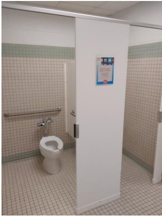
013011a 1/11/2023 Nonaccessible water closet Room 3601
