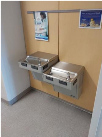
013025a 1/11/2023 Typical dual height water fountain Room 3006
