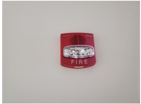
013020e 1/11/2023 Fire alarm system notifier Corridor 3004
