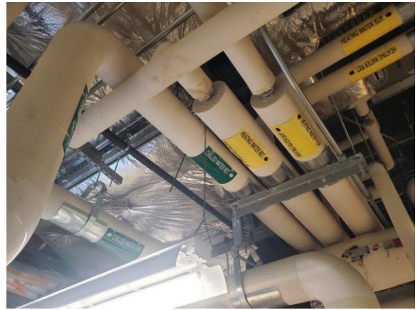
013052e 1/11/2023 Overview of various systems Room 1307
