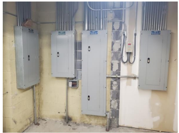
013015e 1/11/2023 Siemens secondary electric panelboards Room 3303
