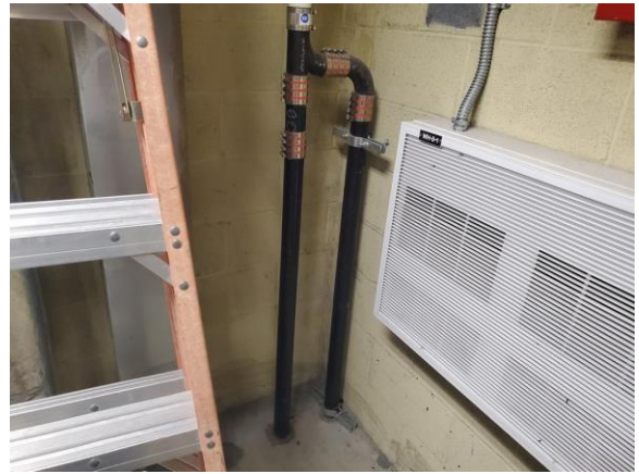
013017e 1/11/2023 ABS waste piping Room 3303
