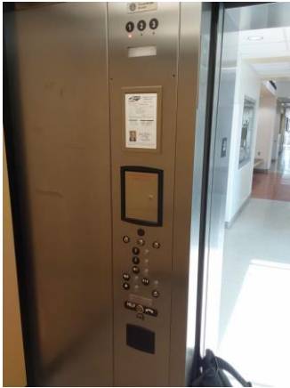
013062a 1/11/2023 Compliant elevator control board Elevator
