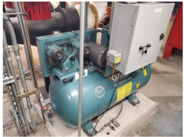
013057e 1/11/2023 HVAC control system air compressor Room 1307
