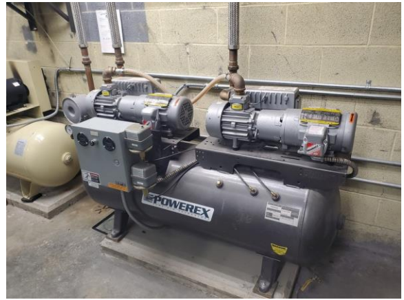
013053e 1/11/2023 Duplex vacuum pump system Room 1307
