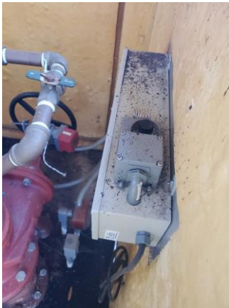
013071e 1/11/2023 Electric heater for fire backflow Exterior
