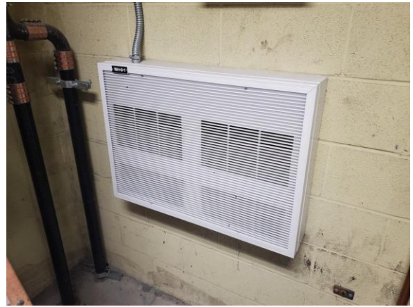
013016e 1/11/2023 Electric unit heater WH-3-1 Room 3303
