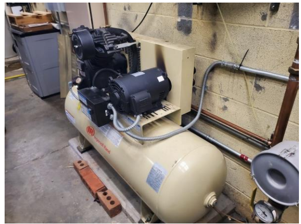
013054e 1/11/2023 Process and lab air compressor Room 1307
