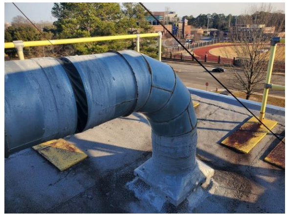
013003e 1/11/2023 Slight corrosion on steel ductwork Roof
