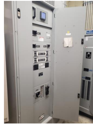
013047e 1/11/2023 Main electrical distribution panelboard Room 1305
