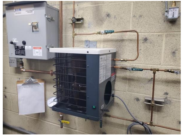
013056e 1/11/2023 Hankison air dryer Room 1307
