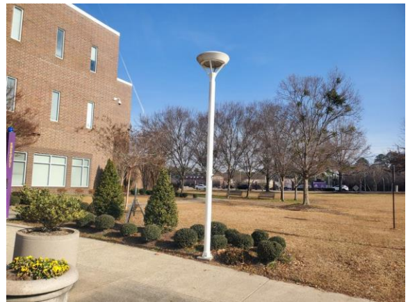
013076e 1/11/2023 Pole-mounted exterior lighting with LED lamp Site
