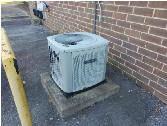
013069e 1/11/2023 Air-cooled condenser CU-1-1 Site
