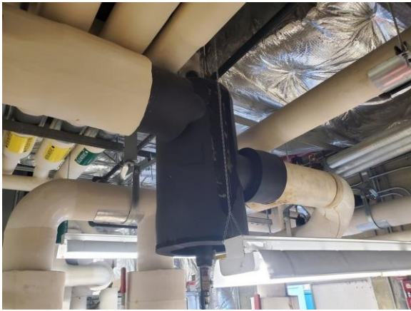
013067e 1/11/2023 Chilled water system air separator Room 1307
