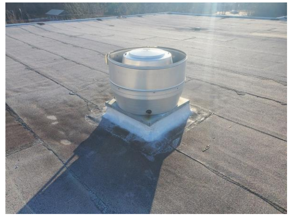
013005e 1/11/2023 General system exhaust fan EF-1-1 Roof
