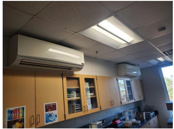
013032e 1/11/2023 Ductless split system blower assemblies Room 3301
