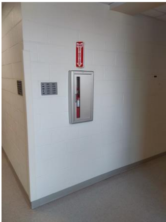
013024a 1/11/2023 Typical fire extinguisher cabinet Room 3004
