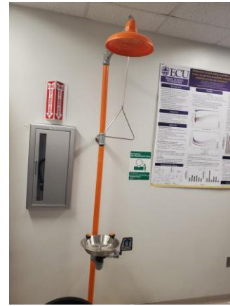
013028e 1/11/2023 Combination safety shower/eyewash station Room 3501
