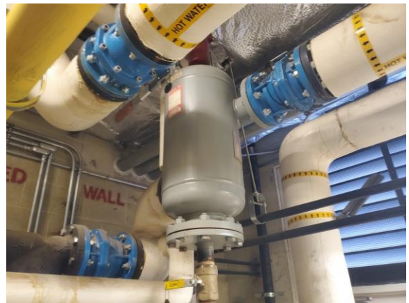
013045e 1/11/2023 Heating water air separator Room 1306
