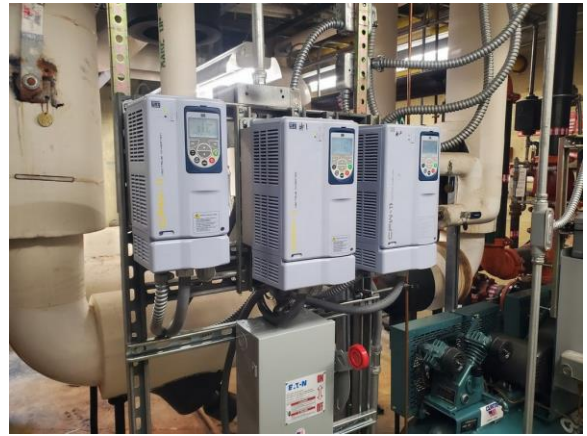
013061e 1/11/2023 Chilled water pump VFDs Room 1307
