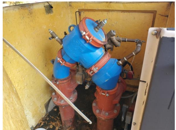
013070e 1/11/2023 Six-inch fire water backflow device Site
