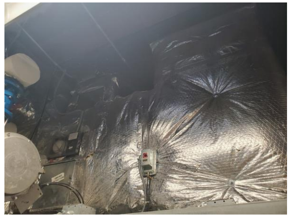
013009e 1/11/2023 Insulated, metal ductwork with detection Room 3303
