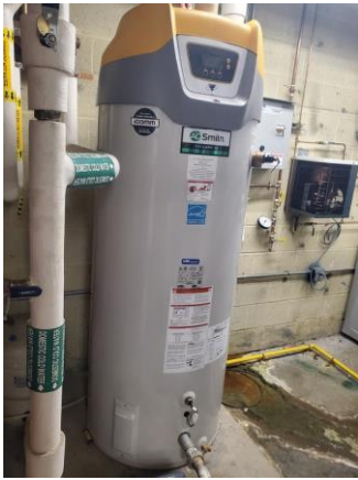
013065e 1/11/2023 Natural gas fired domestic water heater Room 1307
