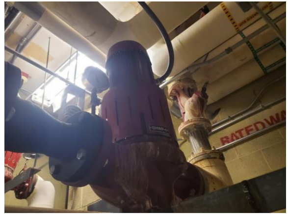
013040e 1/11/2023 Secondary heating water pump SHWP-1 Room 1306
