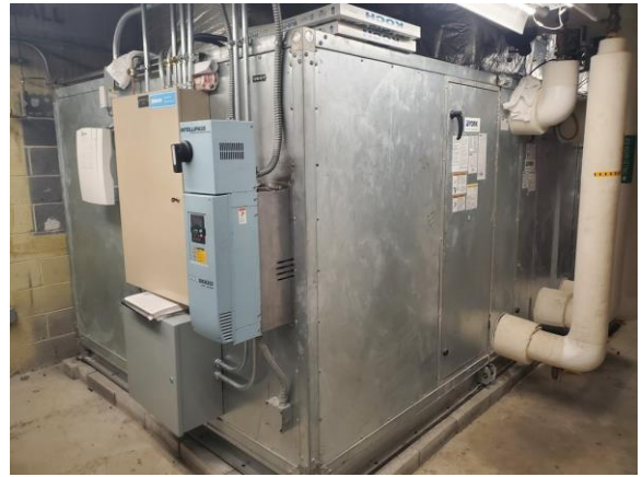
013007e 1/11/2023 Air handler AHU-3-1 Room 3303
