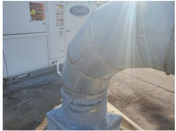
013002e 1/11/2023 Slight corrosion on steel ductwork Roof
