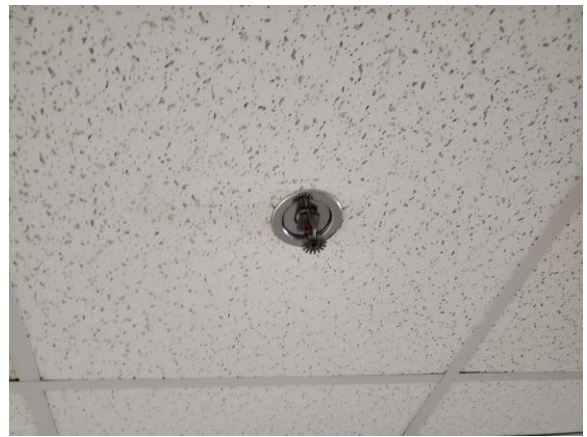
013021e 1/11/2023 Fire suppression system sprinkler head Corridor 3004
