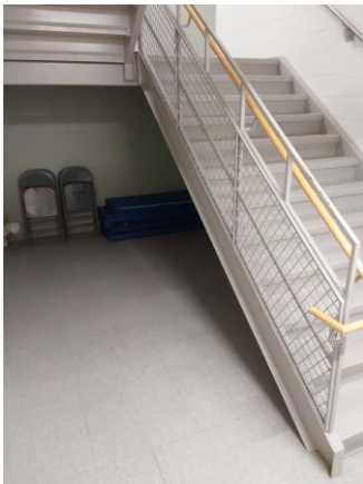
013059a 1/11/2023 Stair tower with missing cane rail Stair 1
