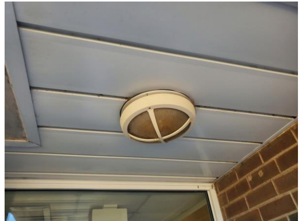
013074e 1/11/2023 Circa 2008 surface mounted HID lighting Exterior
