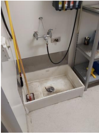
013022a 1/11/2023 Custodial mop sink Room 3307
