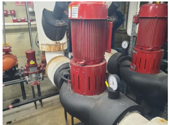
013059e 1/11/2023 Secondary chilled water pumps Room 1307
