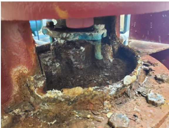
013063e 1/11/2023 Corrosion on fire pump casing Room 1307
