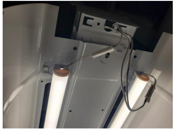
013011e 1/11/2023 LED retrofit kit Room 3303
