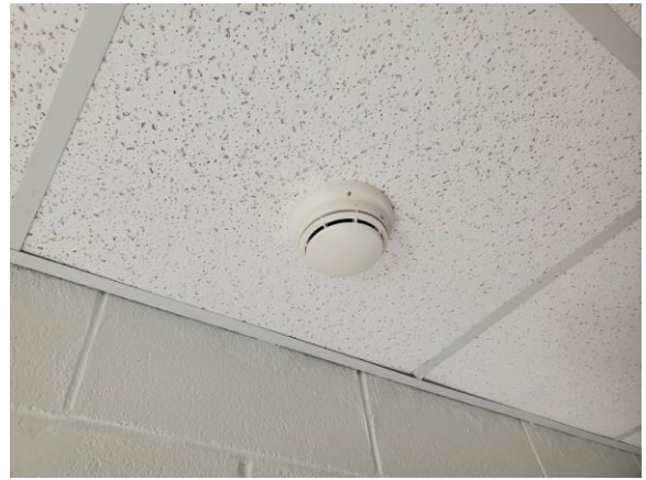
013034e 1/11/2023 Fire alarm system detector Second floor corridor
