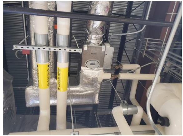
013055e 1/11/2023 Variable air volume terminal unit Room 1307
