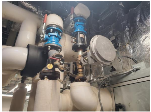
013008e 1/11/2023 Various distribution equipment Room 3303
