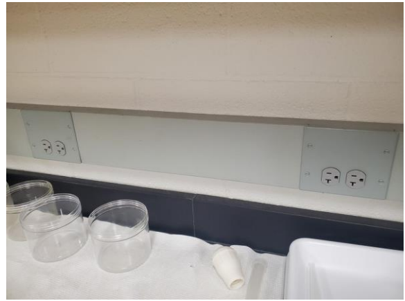
013025e 1/11/2023 Typical electrical outlets Room 3504
