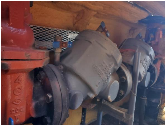
013073e 1/11/2023 Four-inch potable water backflow device Exterior
