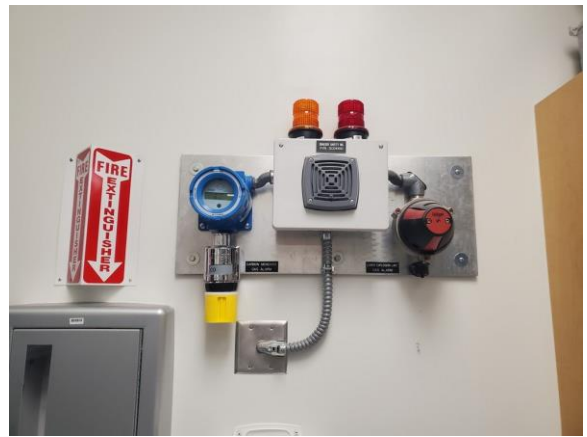
013024e 1/11/2023 Carbon monoxide monitoring system Room 3504
