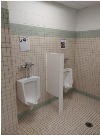
013010a 1/11/2023 Men's urinals Room 3601
