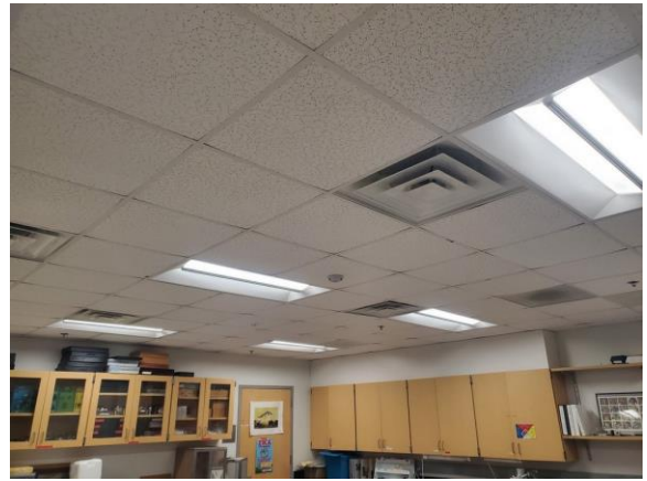
013022e 1/11/2023 Lab/classroom lighting with occupancy Room 3504
