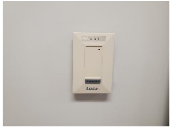
013026e 1/11/2023 Original thermostat for VAV terminal unit Room 3504
