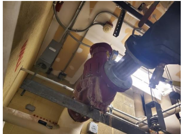
013044e 1/11/2023 Primary heating water pump PHWP-1 Room 1306
