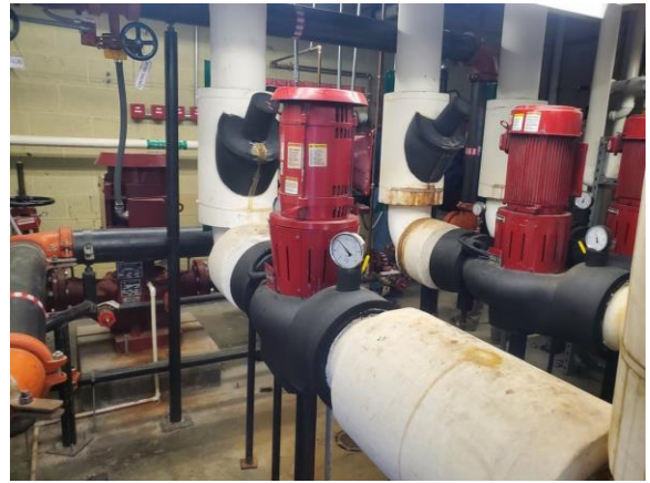
013058e 1/11/2023 Primary chilled water pump Room 1307
