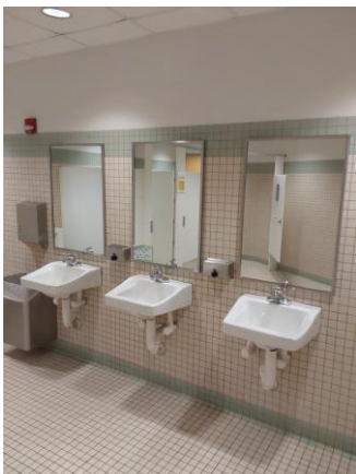
013042a 1/11/2023 Wall-hung lavatories Room 1602
