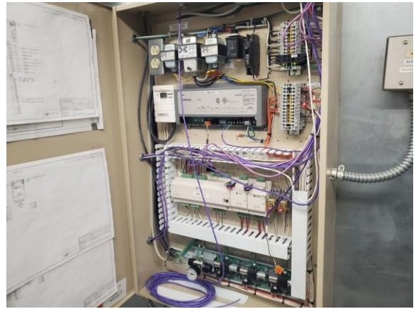
013013e 1/11/2023 DDC control panel CP-3-1 with updates Room 3303
