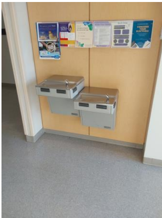
013033a 1/11/2023 Dual-height water fountain Room 2001
