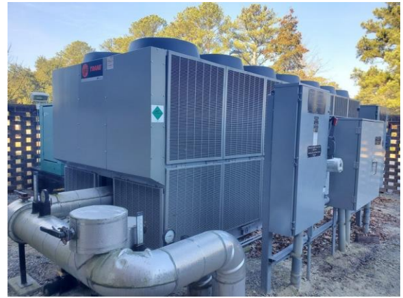
013049e 1/11/2023 Updated air-cooled chiller Site
