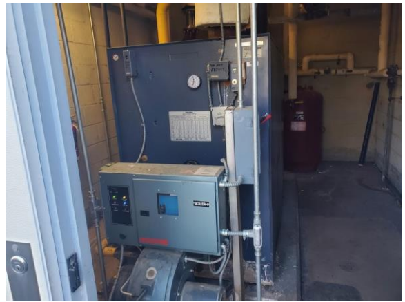
013039e 1/11/2023 Natural gas heating water boiler Room 1306
