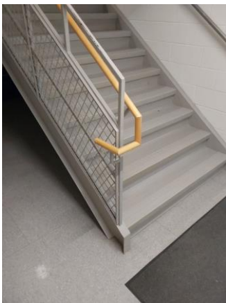
013060a 1/11/2023 Stair tower with missing handrail extension Stair 1
