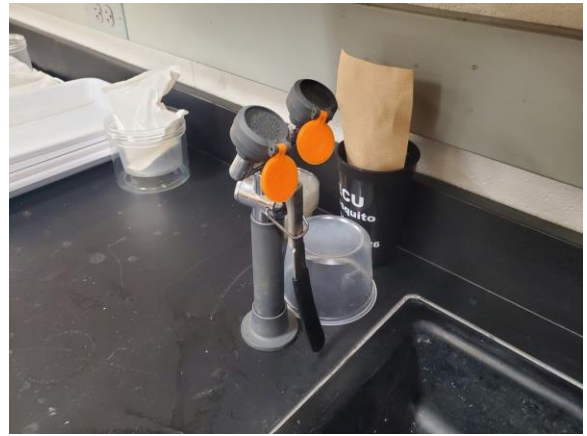
013023e 1/11/2023 Eyewash/drench hose Room 3504
