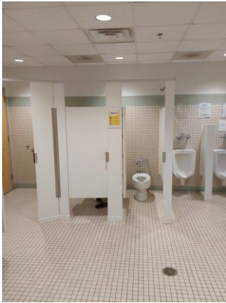
013041a 1/11/2023 Urinals, water closet, partitions, and ceramic wall and floor tile Room 1602
