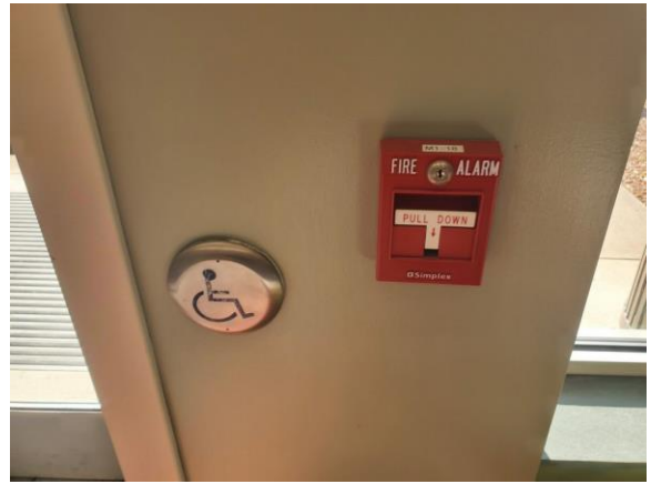
013037e 1/11/2023 Fire alarm system pull station Vestibule 1002
