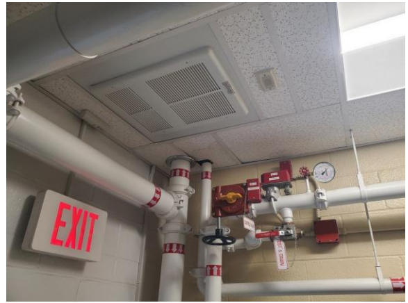
013035e 1/11/2023 Fire riser, tamper switches, flow switches Stair S-2
