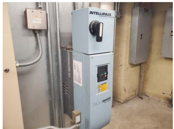
013012e 1/11/2023 Variable speed drive for AHU-3-1 supply fan Room 3303
