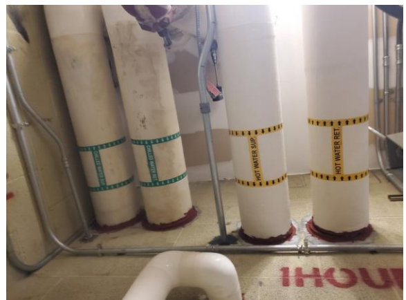
013042e 1/11/2023 Primary heating and chilled water pipe Room 1306
