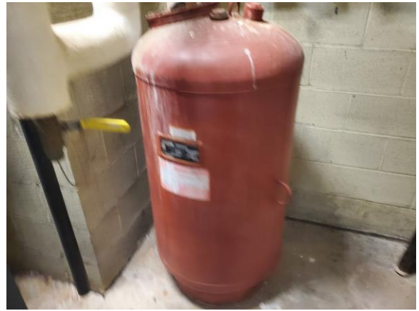
013041e 1/11/2023 Heating water expansion tank Room 1306
