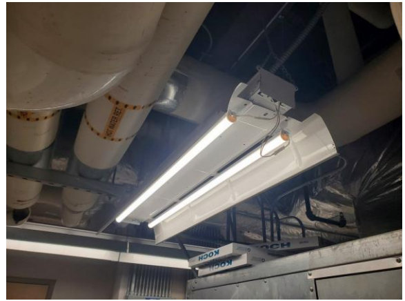
013010e 1/11/2023 Pendant style lighting with LED retrofit kit Room 3303
