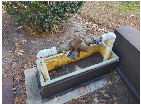
013072e 1/11/2023 Irrigation water backflow Site
