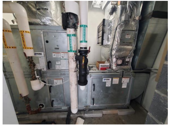
013031e 1/11/2023 Air handler AHU-3-2 for computer lab Room 3101
