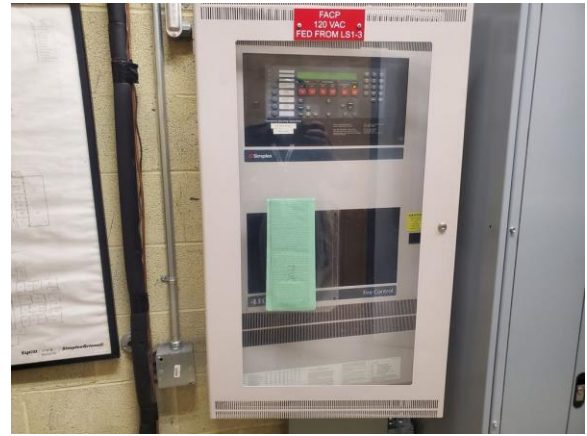
013046e 1/11/2023 Fire alarm control panel Room 1305
