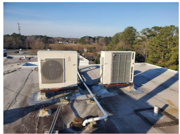
013006e 1/11/2023 Ductless split system air-cooled condensers Roof
