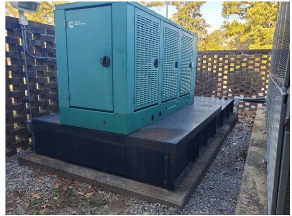
013050e 1/11/2023 Diesel fired emergency generator Site
