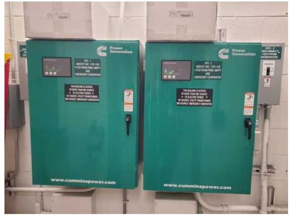
013038e 1/11/2023 Two automatic transfer switches Room 1303
