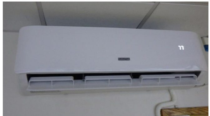
164030e 1/25/2023 Split ductless evaporator Command center 138
