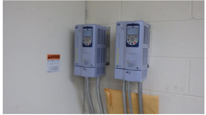
164028e 1/25/2023 Chilled water pump P-1 and P-2 VFDs Server 144
