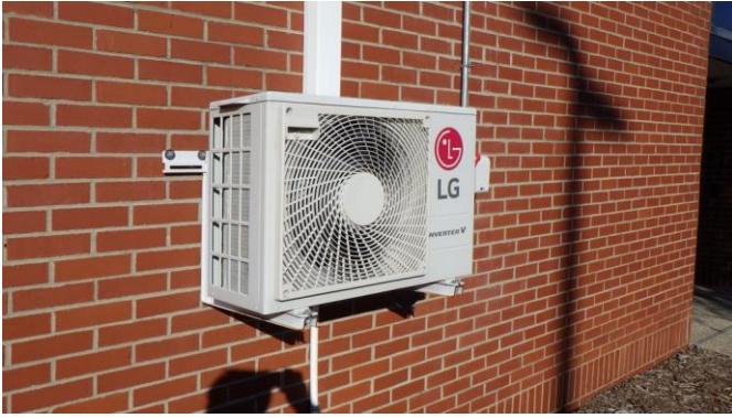
164076e 1/25/2023 Split ductless system air-cooled condenser South elevation
