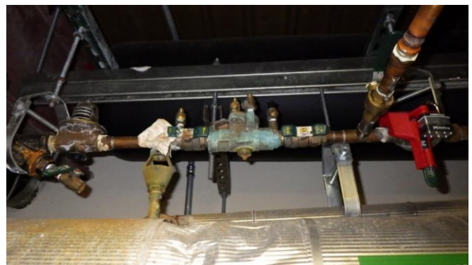
164039e 1/25/2023 Domestic water backflow preventer Mechanical 0136A
