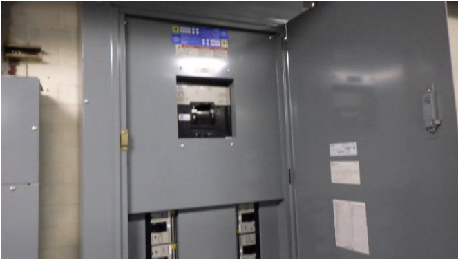
164058e 1/25/2023 Main electrical distribution panel DP Electrical 137
