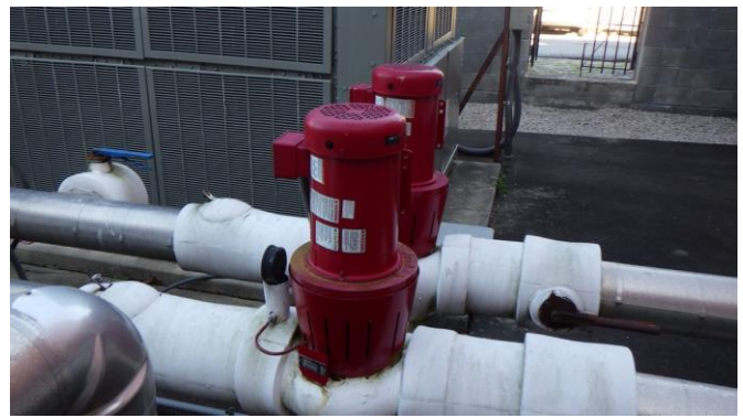
164073e 1/25/2023 Chilled water pumps P-1 and P-2 North elevation
