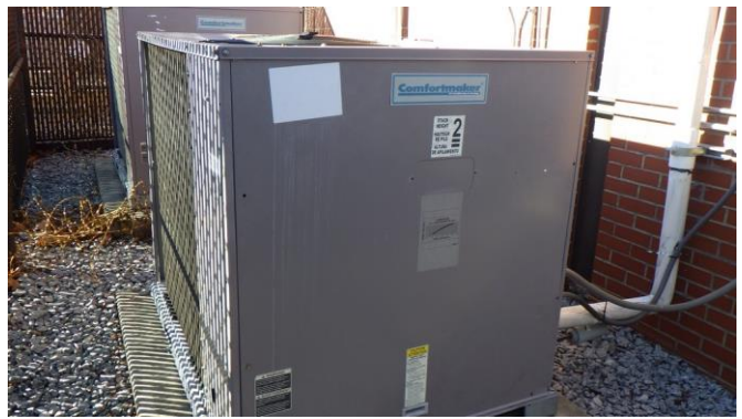
164067e 1/25/2023 Air-cooled condensing units Southeast corner
