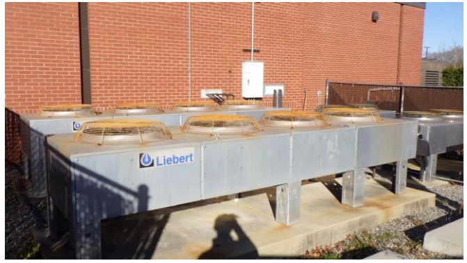
164077e 1/25/2023 Liebert CRAC unit air-cooled condensers South elevation
