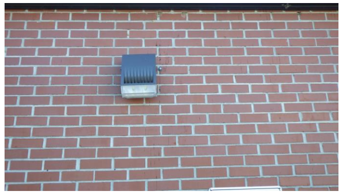
164061e 1/25/2023 LED wall pack East side
