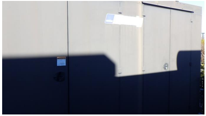
164065e 1/25/2023 Diesel-fueled emergency generator 1 East side
