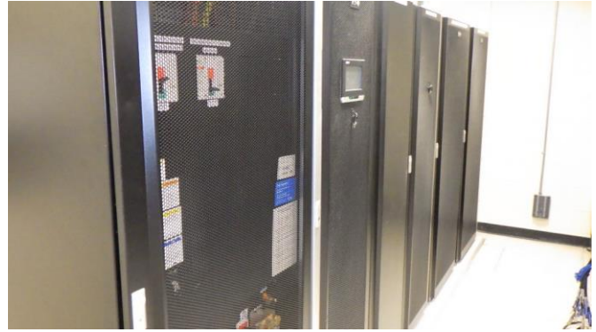
164031e 1/25/2023 UPS-1 Server room 133
