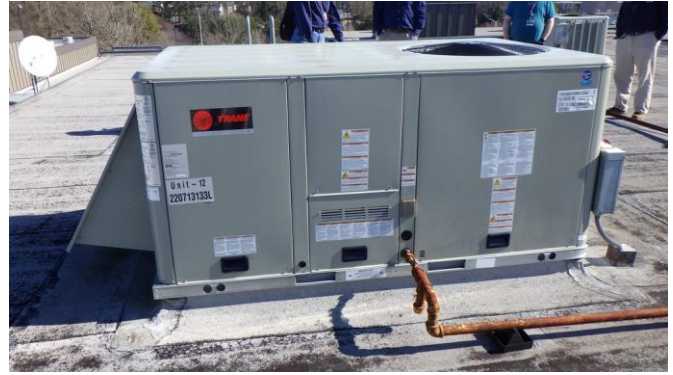
164010e 1/25/2023 Rooftop package unit GP-12 Roof
