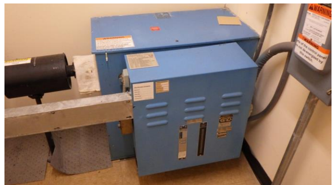
164018e 1/25/2023 Hydraulic elevator machine Elevator 0219
