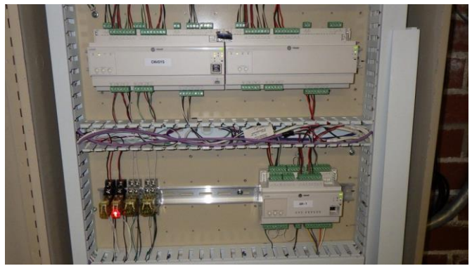
164043e 1/25/2023 HVAC DDC controls Mechanical 0136A
