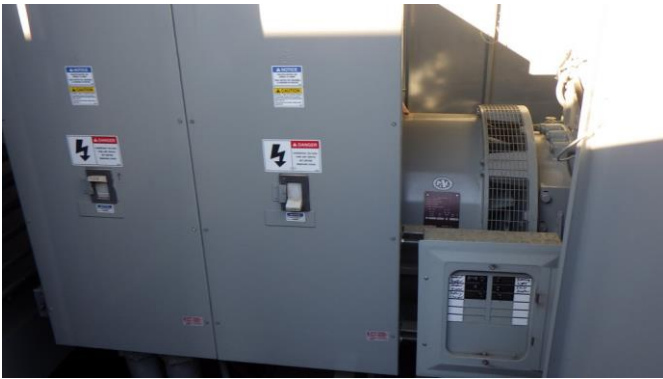
164066e 1/25/2023 Diesel-fueled emergency generator Generator 1
