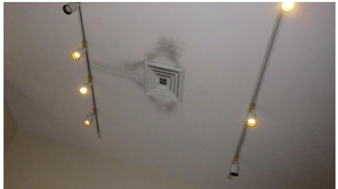
164008e 1/25/2023 Central HVAC distribution grill (mildew) Lobby 0101
