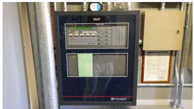
164051e 1/25/2023 Main fire alarm control panel Electrical 137
