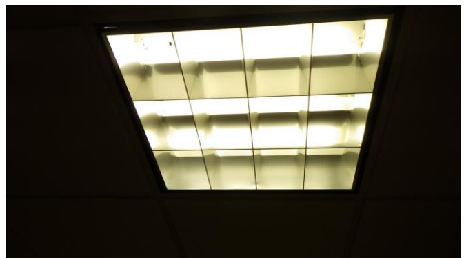
164006e 1/25/2023 Open parabolic lay-in fluorescent interior light fixture Conference 0161
