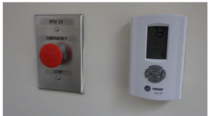
164015e 1/25/2023 HVAC digital thermostat and emergency power kill switch Open office 0223
