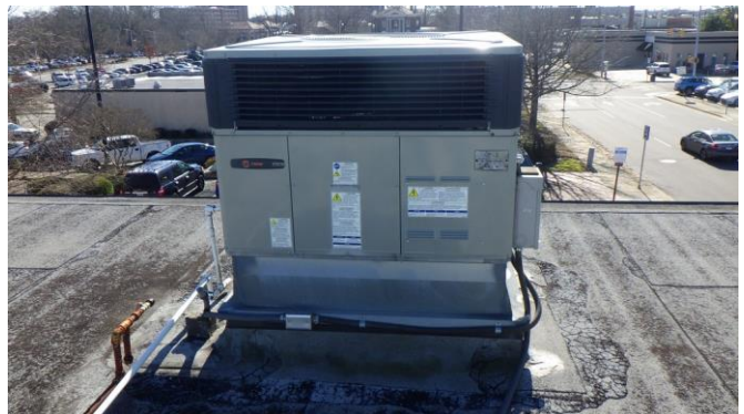
164009e 1/25/2023 Rooftop package unit GP-2 Roof
