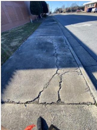
164023a 1/25/2023 Broken sidewalk Exterior
