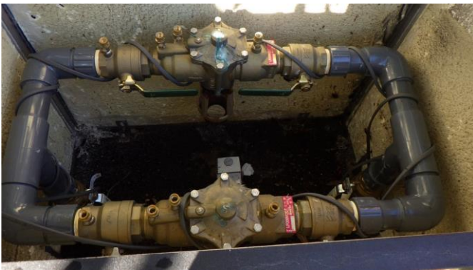
164074e 1/25/2023 Cooling water backflow preventers South elevation
