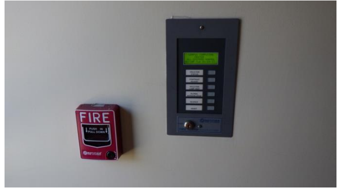
164001e 1/25/2023 Annunciator panel and manual pull station Lobby 0101
