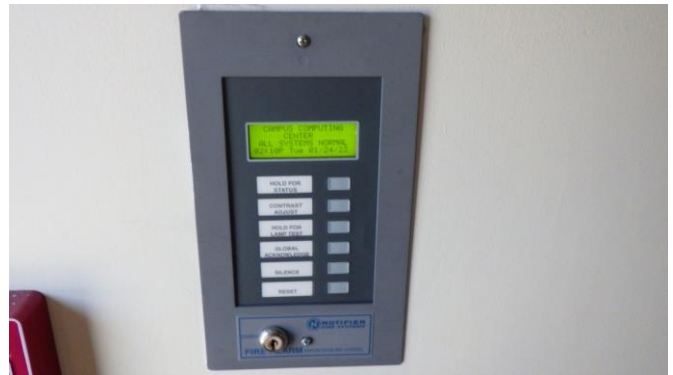
164002e 1/25/2023 Annunciator panel Lobby 0101
