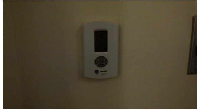
164004e 1/25/2023 HVAC digital thermostat Lobby 0101
