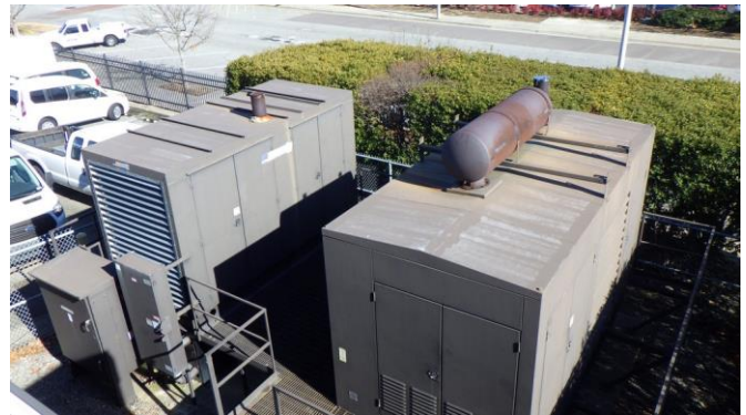
164014e 1/25/2023 Emergency generators North elevation
