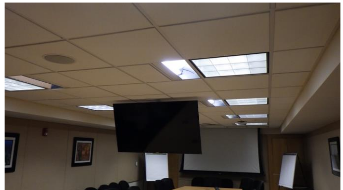
164024e 1/25/2023 Open parabolic lay-in fluorescent interior light fixtures Conference 0108
