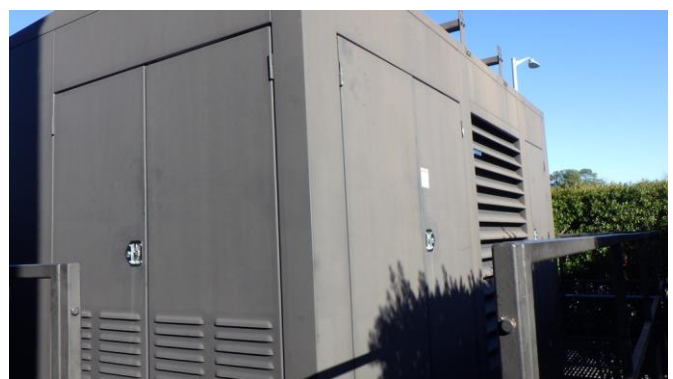
164063e 1/25/2023 Diesel-fueled emergency generator 2 East side
