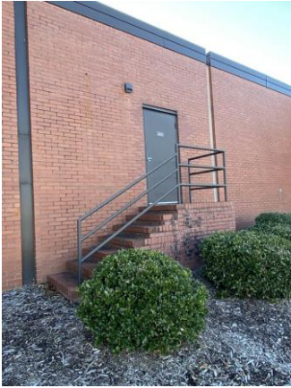
164025a 1/25/2023 Brick exterior, metal door, and stairs with lack and of wall handrail and noncompliant handrails Exterior
