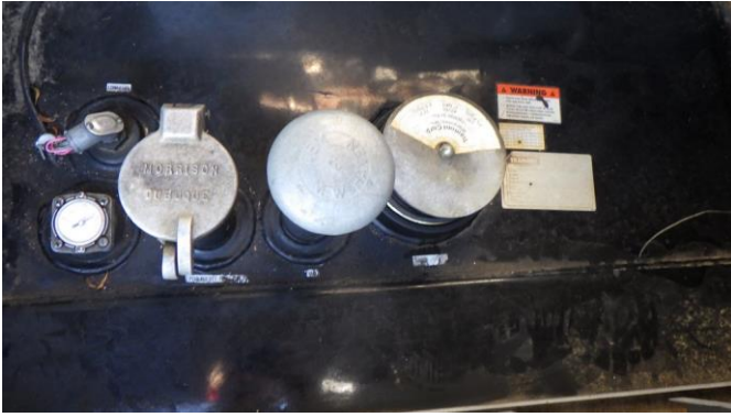
164064e 1/25/2023 Emergency generator fuel tank fill ports Generator 2
