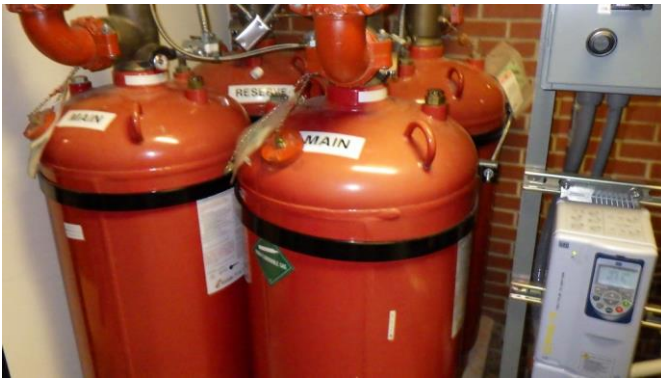
164036e 1/25/2023 FM 200 fire suppression storage tanks Mechanical 0136A
