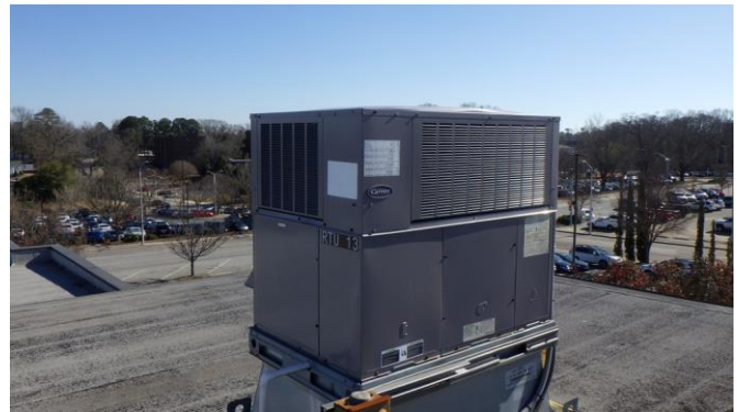
164011e 1/25/2023 Rooftop package unit GP-13 Roof
