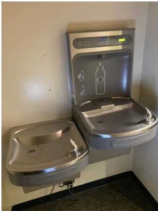
164022a 1/25/2023 Dual-level drinking fountain Corridor
