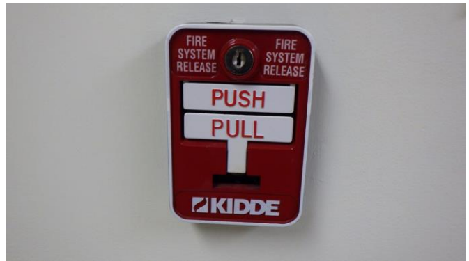
164029e 1/25/2023 Manual pull station Server 140
