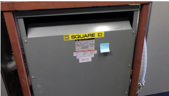
164050e 1/25/2023 Secondary electrical distribution step down transformer Electrical 137
