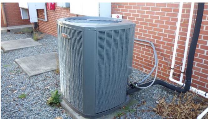
164062e 1/25/2023 Split system air-cooled condenser East side
