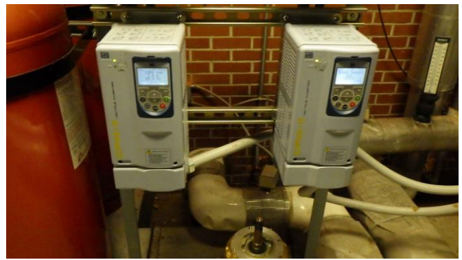
164037e 1/25/2023 Chilled water pump P-3 and P-4 VFDs Mechanical 0136A
