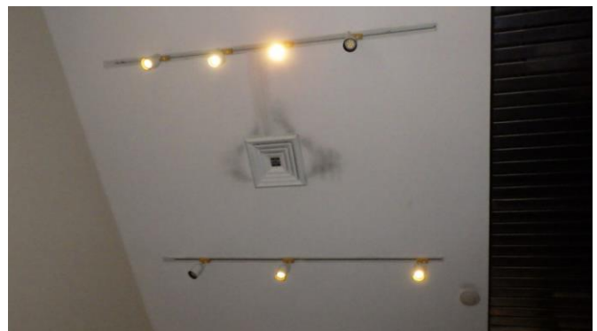
164003e 1/25/2023 Central HVAC distribution grill (mildew) Lobby 0101
