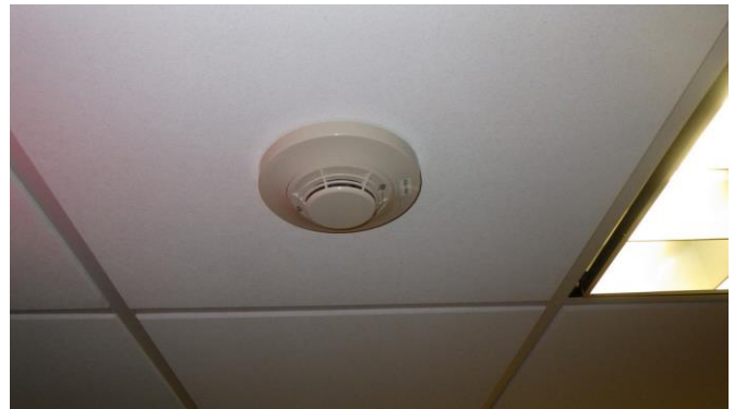
164020e 1/25/2023 Smoke detector Corridor 0218
