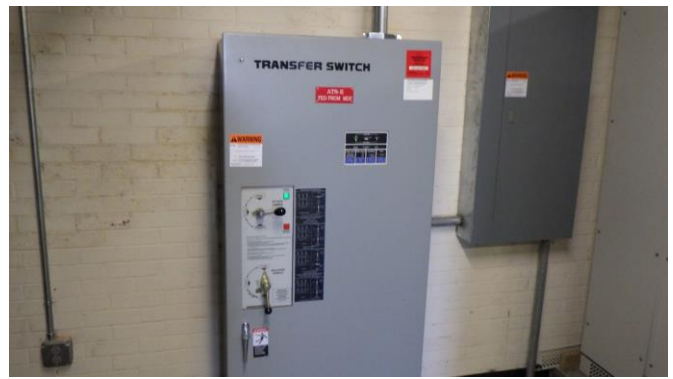
164049e 1/25/2023 Emergency power ATS-E Electrical 137
