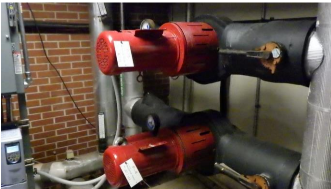
164038e 1/25/2023 Chilled water pumps P-3 and P-4 Mechanical 0136A
