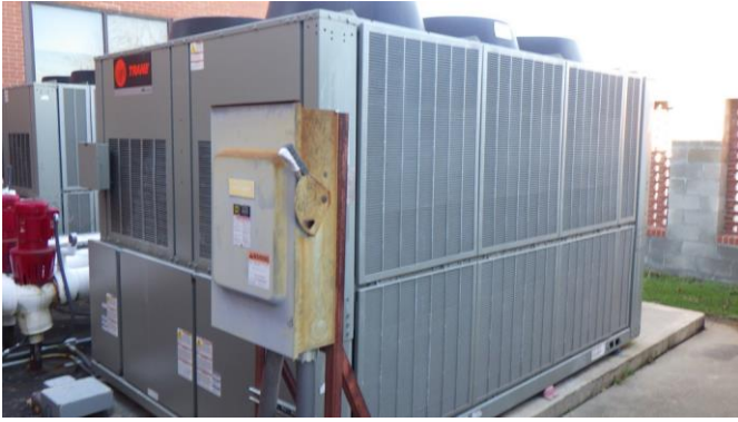
164070e 1/25/2023 Air-cooled chiller CH-1 North elevation
