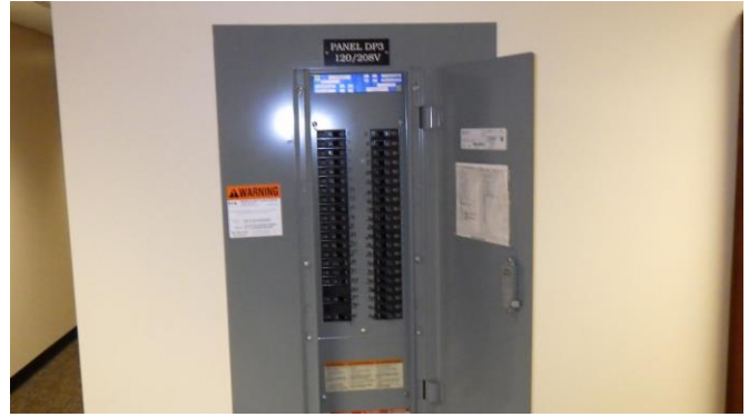
164019e 1/25/2023 Secondary electrical distribution panel DP3 Corridor 0218
