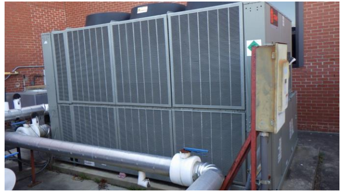
164071e 1/25/2023 Air-cooled chiller CH-2 North elevation
