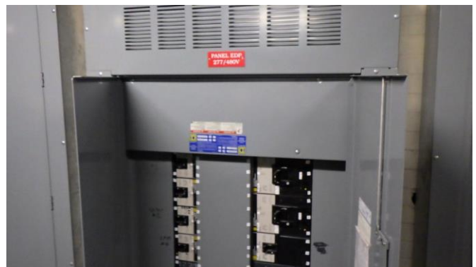
164057e 1/25/2023 Emergency power electrical distribution panel EDP Electrical 137
