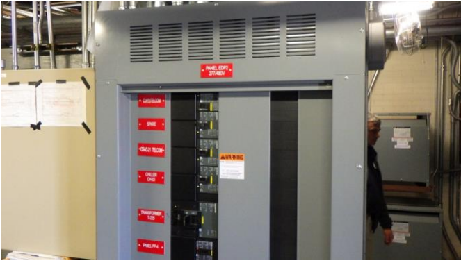
164052e 1/25/2023 Emergency power electrical distribution panel EDP2 Electrical 137
