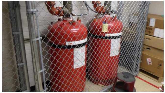
164035e 1/25/2023 FM 200 fire suppression storage tanks Shipping and receiving 0136
