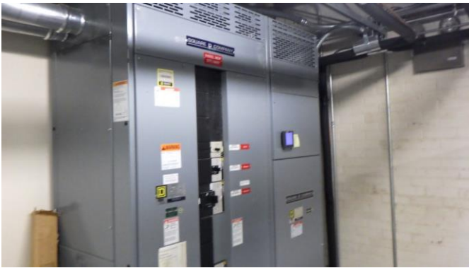
164048e 1/25/2023 Main electrical distribution panel MDP Electrical 137
