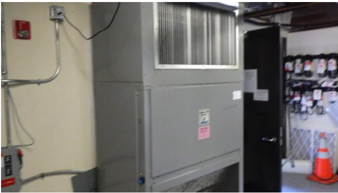
164060e 1/25/2023 AC package unit AC-1 Electrical 137
