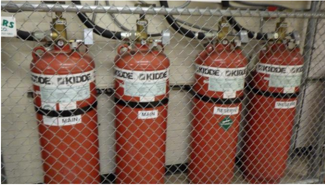
164034e 1/25/2023 FM 200 fire suppression storage tanks Shipping and receiving 0136
