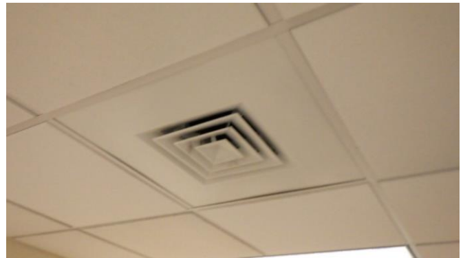
164017e 1/25/2023 Central HVAC distribution grill Open office 0223
