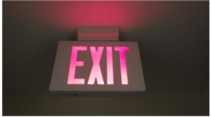
164007e 1/25/2023 Illuminated emergency exit sign Corridor 0159
