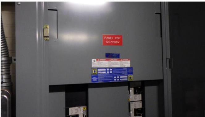
164056e 1/25/2023 Main electrical distribution panel CDP Electrical 137
