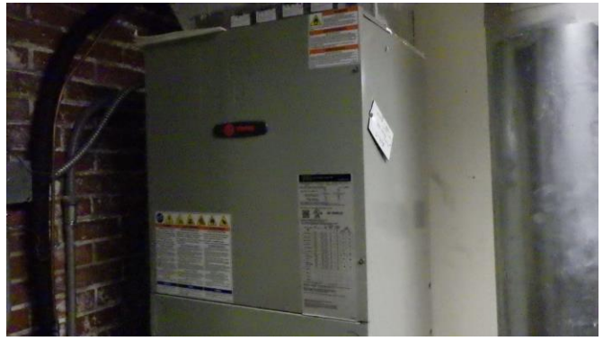
164041e 1/25/2023 Indoor air handler AH-1 Mechanical 0136A
