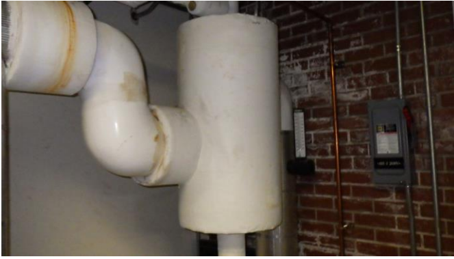
164040e 1/25/2023 Chilled water distribution network expansion tank Mechanical 0136A
