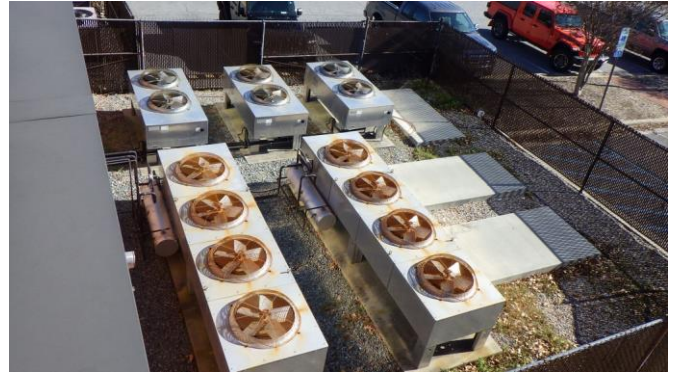
164013e 1/25/2023 Condensing racks for computer room ACs Northeast corner
