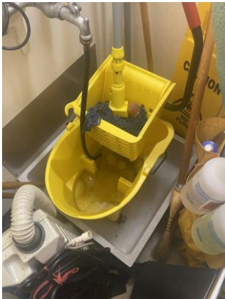
164008a 1/25/2023 Composite utility sink Custodial room
