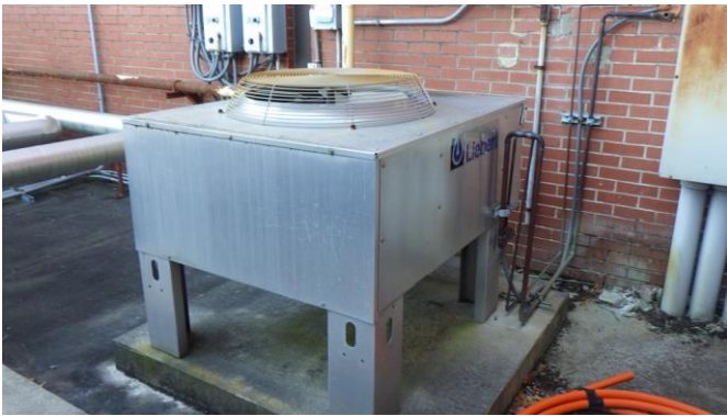
164072e 1/25/2023 Liebert CRAC unit air-cooled condenser North elevation
