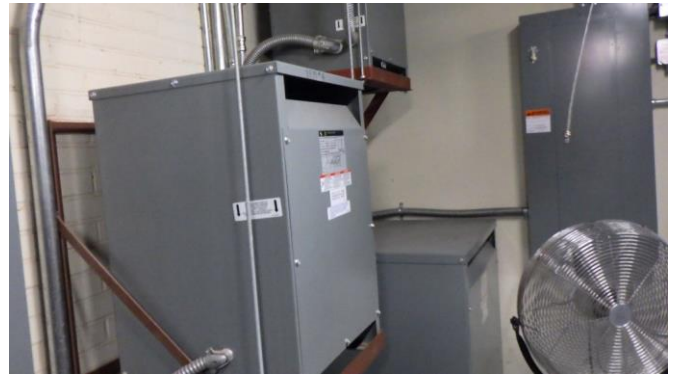
164059e 1/25/2023 Secondary electrical distribution step down transformers Electrical 137
