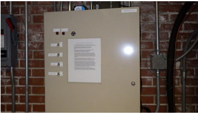
164042e 1/25/2023 HVAC DDC controls cabinet Mechanical 0136A
