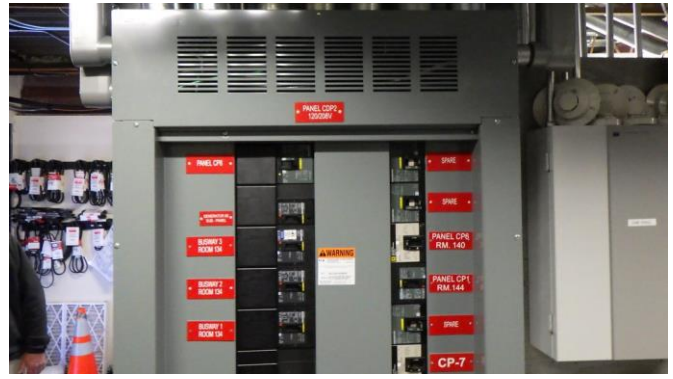
164053e 1/25/2023 Main electrical distribution panel CDP2 Electrical 137
