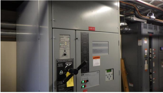
164046e 1/25/2023 Emergency power ATS-B Electrical 137
