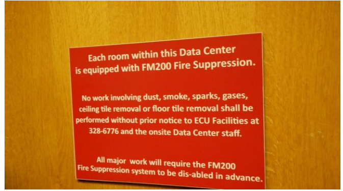
164025e 1/25/2023 FM 200 fire suppression warning sign Telecom 145
