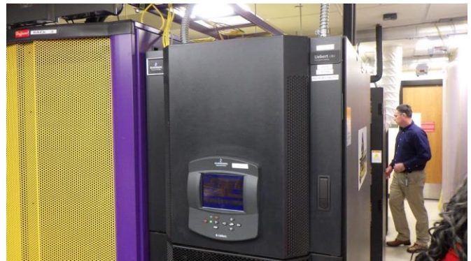
164033e 1/25/2023 Server rack cooling CRV-3 Server room 133
