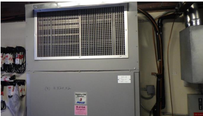
164044e 1/25/2023 AC package unit AC-2 Electrical 137
