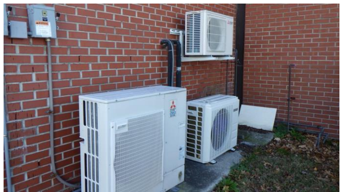
164069e 1/25/2023 Split ductless system air-cooled condensers North elevation
