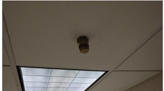
164026e 1/25/2023 FM 200 fire suppression nozzle Telecom 145
