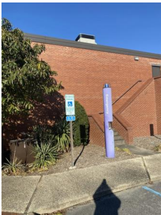
164033a 1/25/2023 Steps lacking handrails Exterior
