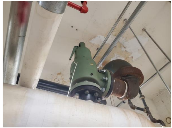
002059e 1/9/2023 Steam safety relief Room 153
