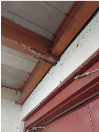
002014a 1/9/2023 Corrosion of structural steel members Roof attic
