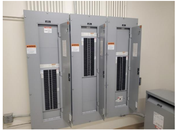
002037e 1/9/2023 Secondary electric panelboards Room 372
