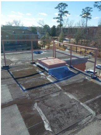
002006a 1/9/2023 Roof hatch with worn fall protection Roof
