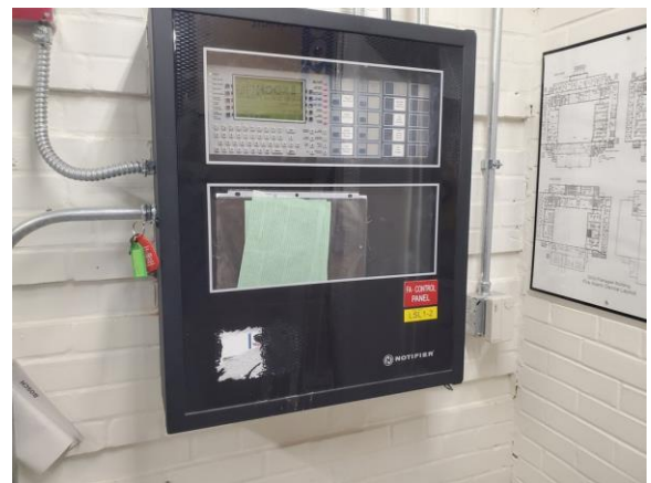
002072e 1/9/2023 Fire alarm control panel Room 105
