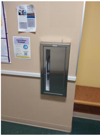
002071a 1/9/2023 Typical fire extinguisher cabinet Room 2202
