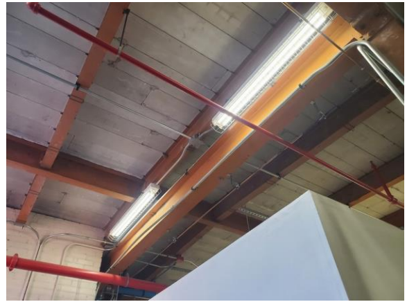
002005e 1/9/2023 Surface-mounted lighting Room 450
