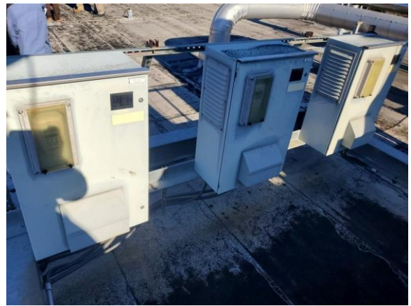
002003e 1/9/2023 Variable speed drives for LEF-1 through LEF-3 Roof
