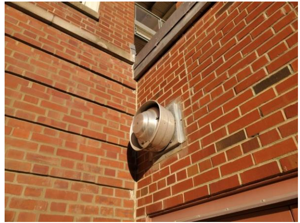
002077e 1/9/2023 Through wall exhaust fan Room 105
