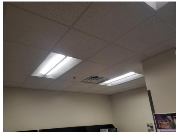
002039e 1/9/2023 2x4 recessed light fixtures with LED retrofit Room 372
