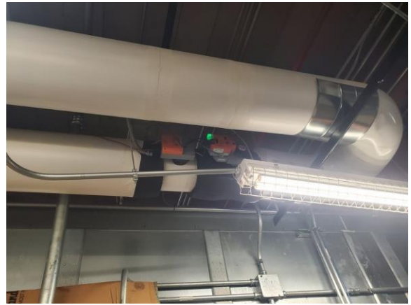
002022e 1/9/2023 Updated control system actuators Room 450
