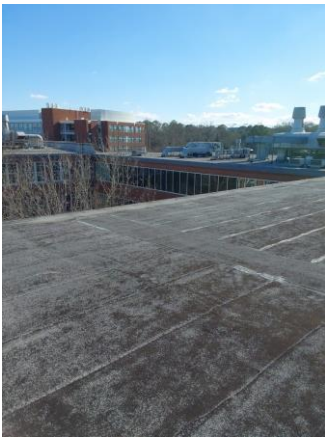
002003a 1/9/2023 Roof edge with no parapet Roof
