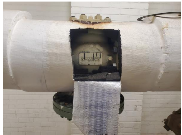
002060e 1/9/2023 Steam pressure reducing station Room 153
