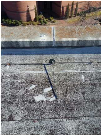
002010a 1/9/2023 Lighting protection system detached from roof Roof
