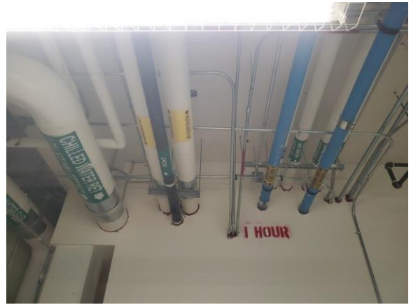
002053e 1/9/2023 Various piping systems Room 2205
