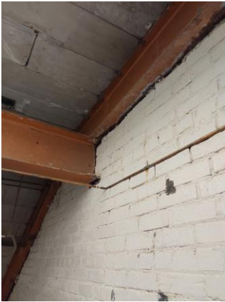
002011a 1/9/2023 Corrosion of structural steel members Roof attic
