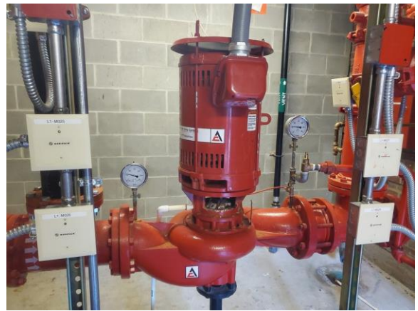
002081e 1/9/2023 Electric fire suppression system pump Room 196
