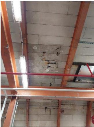
002018a 1/9/2023 Signs of water damage Roof attic
