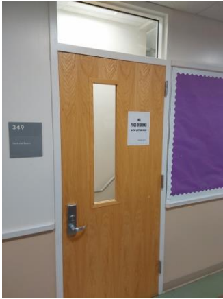
002034a 1/9/2023 Fire-rated door with rated glass Room 349
