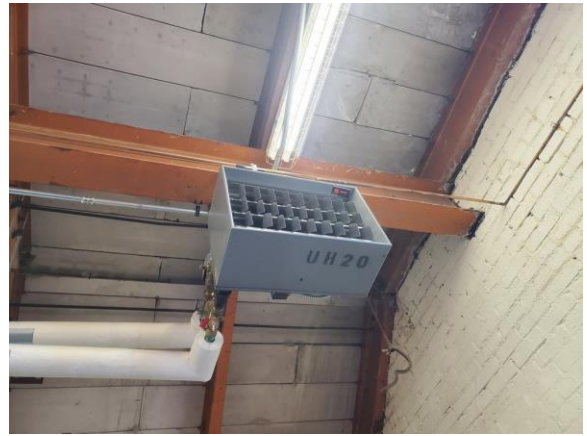
002007e 1/9/2023 Hydronic unit heater UH-20 Room 450
