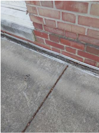
002102a 1/9/2023 Concrete backer against brick has deteriorated West elevation
