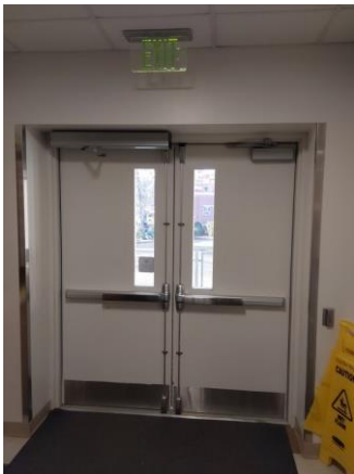
002069a 1/9/2023 Doors with power door operator Room 2202
