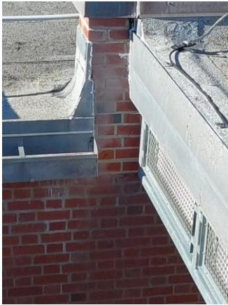
002007a 1/9/2023 Cracked brick above gutter Roof
