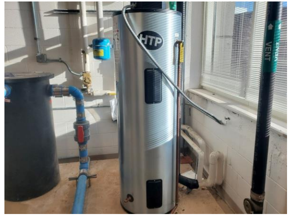
002052e 1/9/2023 Electric water heater Room 2205
