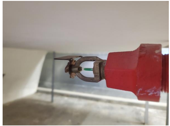
002008e 1/9/2023 Sprinkler head Room 450
