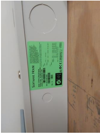
002046a 1/9/2023 Door access box third floor Room 370
