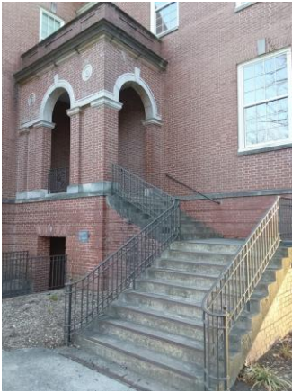
002100a 1/9/2023 Noncompliant stair rail Northwest elevation
