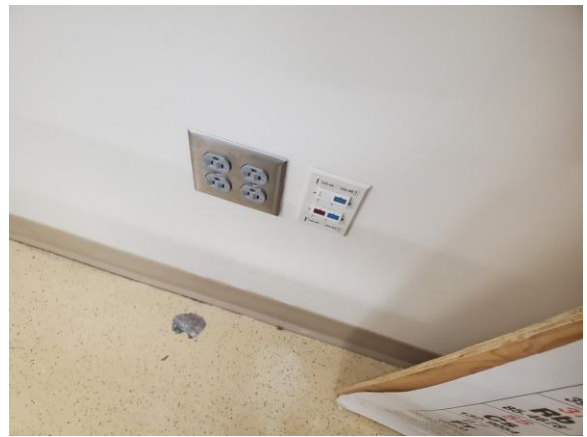
002036e 1/9/2023 Typical electrical outlet and CAT connection Room 372
