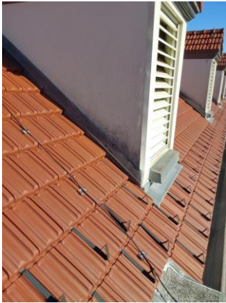
002004a 1/9/2023 Grime on EIFS siding of dormers Roof
