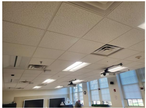
002030e 1/9/2023 Overview of computer lab systems Room 337
