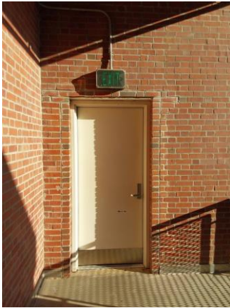
002058a 1/9/2023 Missing panic hardware Stair 2, 3201
