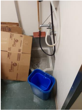
002064a 1/9/2023 Typical mop sink Room 330
