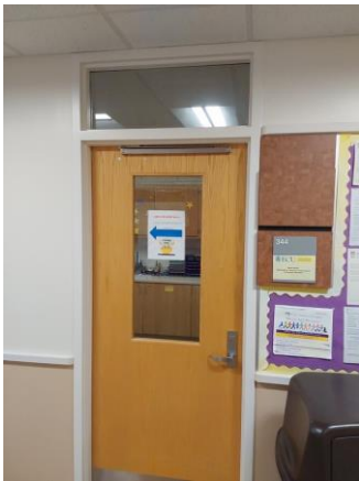
002033a 1/9/2023 Nonrated safety tempered glass on doors Room 340
