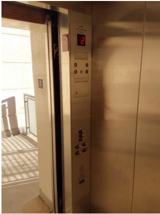
002068a 1/9/2023 Freight elevator control panel Room 214
