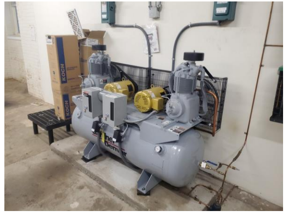
002065e 1/9/2023 Updated pneumatic control air compressor Room 153
