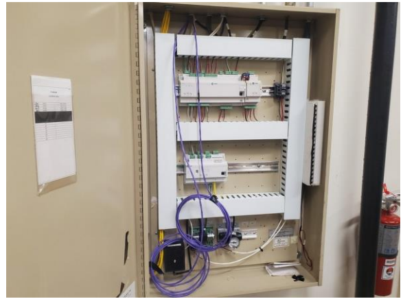
002067e 1/9/2023 Updated HVAC system control panelboard Room 153
