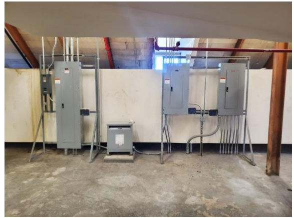
002010e 1/9/2023 Various secondary electrical Room 450
