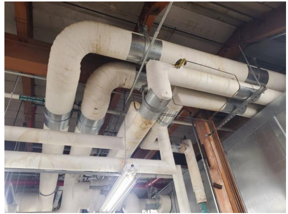
002020e 1/9/2023 Various system piping Room 450
