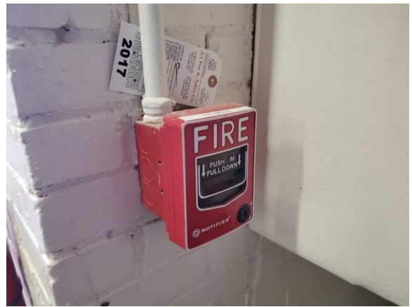
002006e 1/9/2023 Fire alarm pull station Room 450
