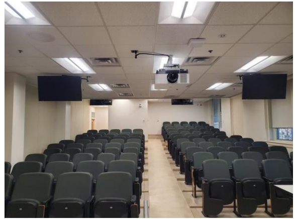
002035e 1/9/2023 Overview of Lecture room systems Room 349
