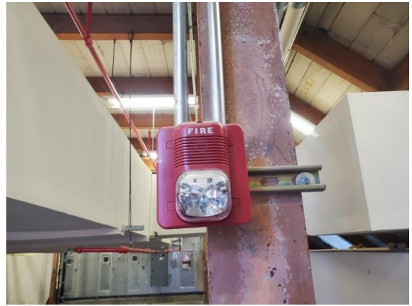
002004e 1/9/2023 Fire alarm system notifier Room 450
