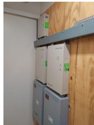
002087a 1/9/2023 Door access control boxes first floor Room 170
