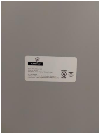
002045a 1/9/2023 Door access control box nameplate Room 370
