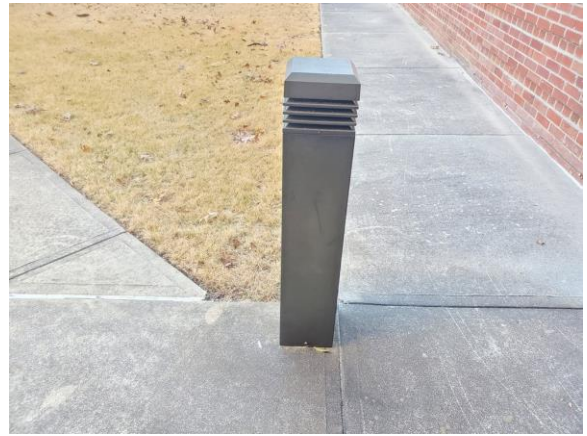
002055e 1/9/2023 Bollard type lighting Courtyard/rock garden
