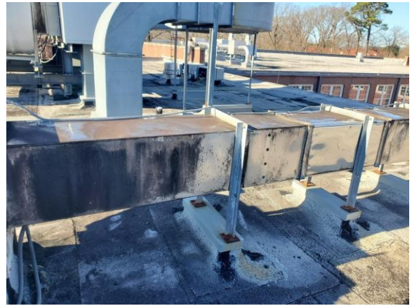
002026e 1/9/2023 Stainless-steel ductwork Roof
