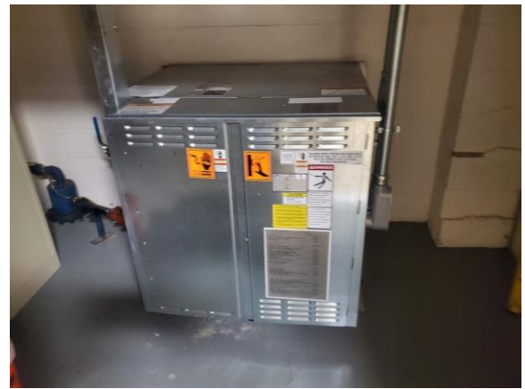
002075e 1/9/2023 Hydraulic elevator machine Room 101
