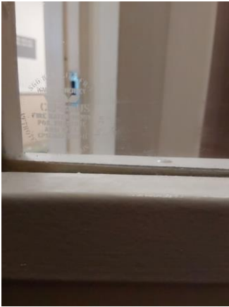
002023a 1/9/2023 Stair tower fire glass rating Stair 3
