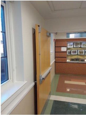
002053a 1/9/2023 Corridor doors with panic hardware Room 340
