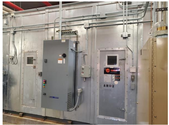
002018e 1/9/2023 Air handler AHU-2 and VFD Room 450
