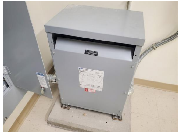
002038e 1/9/2023 Dry-type transformer Room 372
