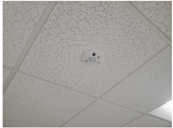
002031e 1/9/2023 Occupancy sensor in computer lab Room 337
