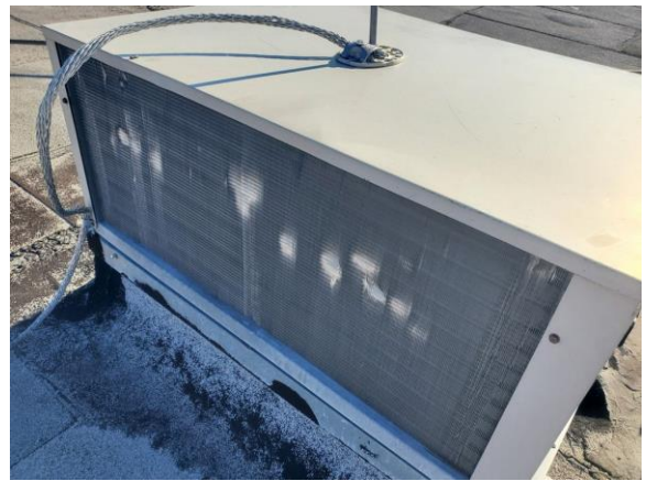
002024e 1/9/2023 Damaged refrigeration unit fin coils Roof
