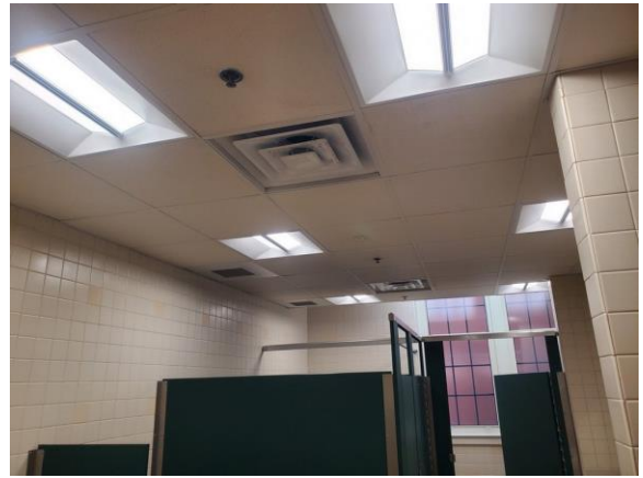
002029e 1/9/2023 Overview of restroom systems Restroom 334
