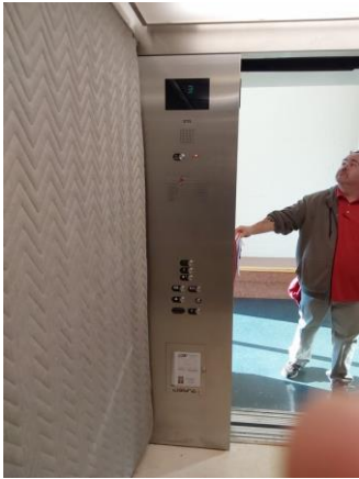
002055a 1/9/2023 Elevator control panel Elevator B
