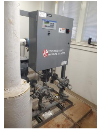
002068e 1/9/2023 Domestic water booster pump system Room 187
