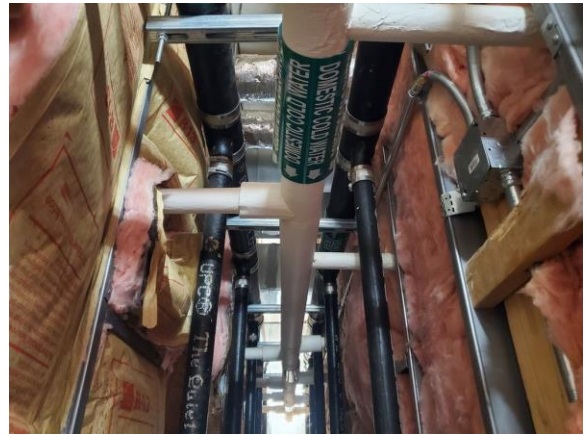
002034e 1/9/2023 Insulated potable water pipe Plumbing chase 336
