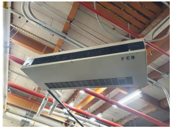
002012e 1/9/2023 Ceiling fan coil FC-9 Room 450
