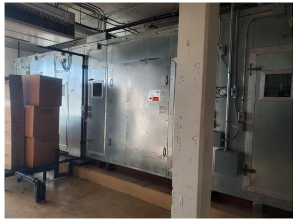
002051e 1/9/2023 Air handler AHU-3 Room 2205
