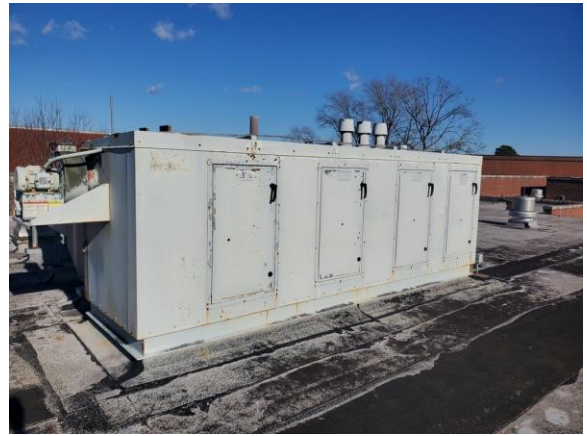
002025e 1/9/2023 Air handler DDU-1 for room 3212 Roof
