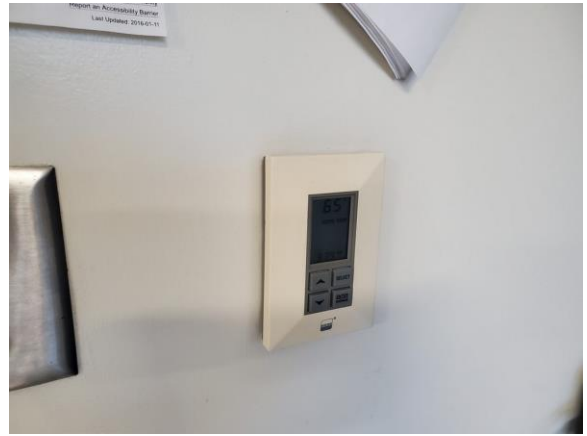
002032e 1/9/2023 Thermostat to be replaced in 2023 Room 337
