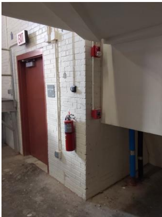
002021a 1/9/2023 Extinguisher with fire pull and alarm Roof attic
