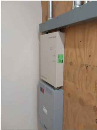
002044a 1/9/2023 Door access control box Room 370
