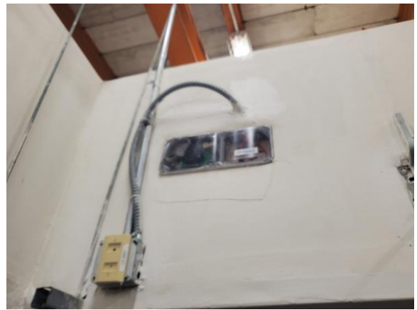
002009e 1/9/2023 HVAC duct work detector Room 450
