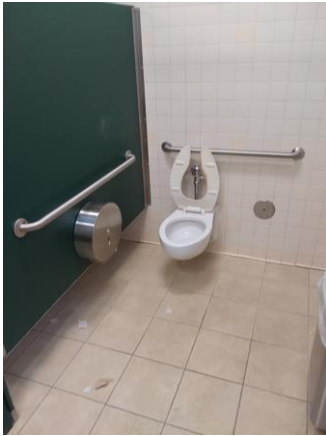
002032a 1/9/2023 ADA toilet and grab bars Room 334
