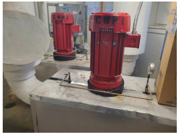
002069e 1/9/2023 Chilled water system pumps Room 187
