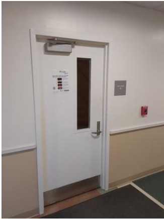
002043a 1/9/2023 Missing panic hardware at Stair tower Stair 4
