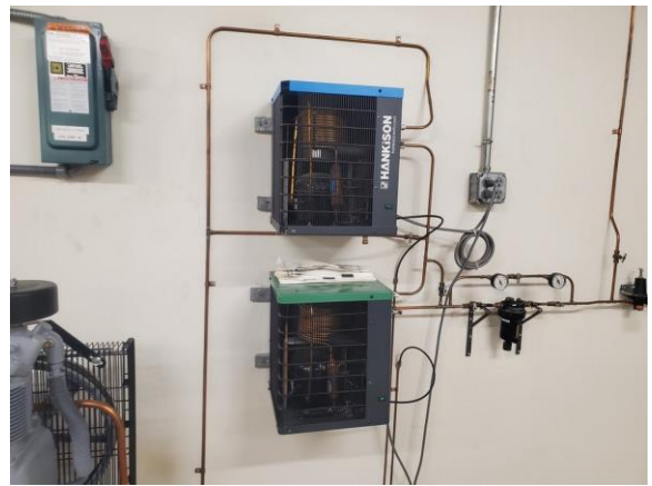
002066e 1/9/2023 Refrigerated air dryers Room 153
