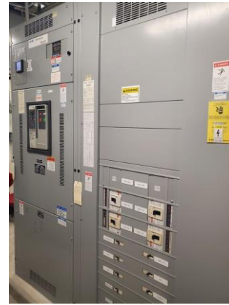
002073e 1/9/2023 1,200-amp MDP and main circuit breaker Room 105
