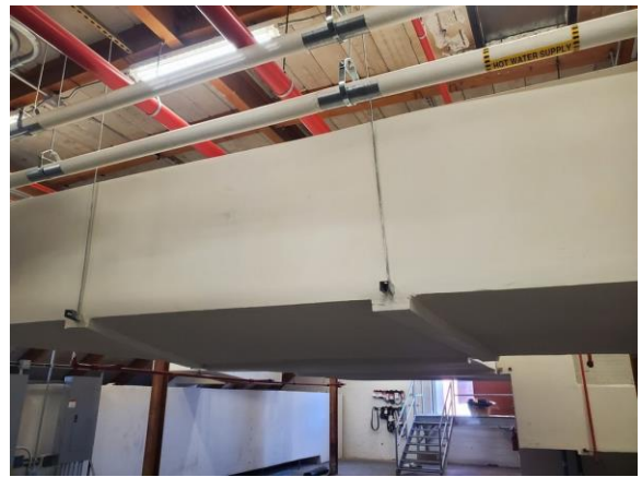
002015e 1/9/2023 Insulated, metal HVAC system ductwork Room 450
