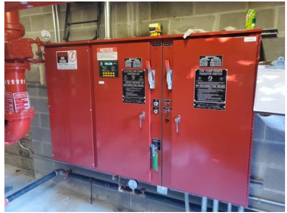
002080e 1/9/2023 Fire pump controller and transfer switch Room 196
