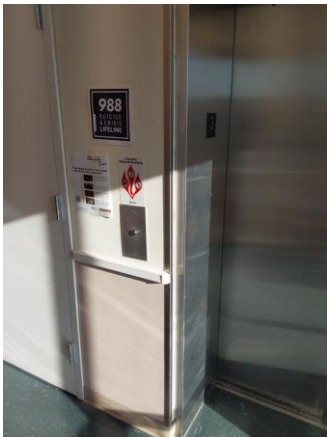
002054a 1/9/2023 Elevator operating button Elevator B
