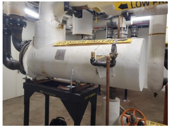
002063e 1/9/2023 Heating water shell-and-tube heat exchanger Room 153
