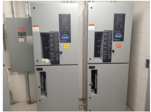
002074e 1/9/2023 Emergency and Life Safety electrical transfer switches Room 105
