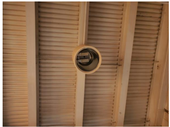
002045e 1/9/2023 Surface mounted exterior lighting Balcony 3201
