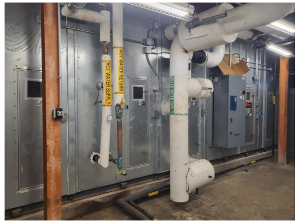
002021e 1/9/2023 Air handler AHU-1 Room 450
