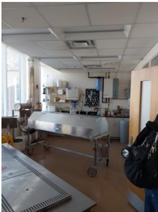
002063a 1/9/2023 Lab with epoxy flooring and damaged ceiling Room 3212
