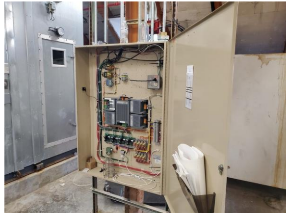
002011e 1/9/2023 HVAC with legacy DDC control equipment Room 450
