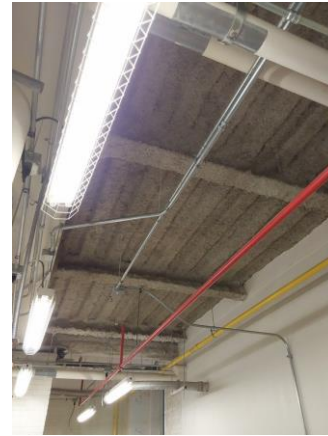
002085a 1/9/2023 Exposed steel fireproofing Room 153
