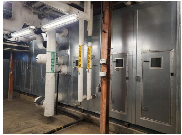
002019e 1/9/2023 Heating and chilled water pipe for AHU-2 coils Room 450
