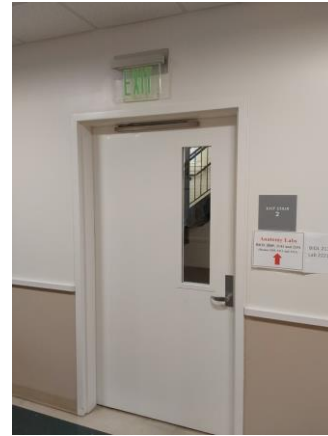
002091a 1/9/2023 Exit door in need of panic hardware Stair 2
