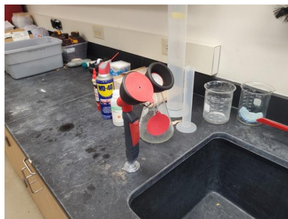
002042e 1/9/2023 Emergency eyewash station Room 382
