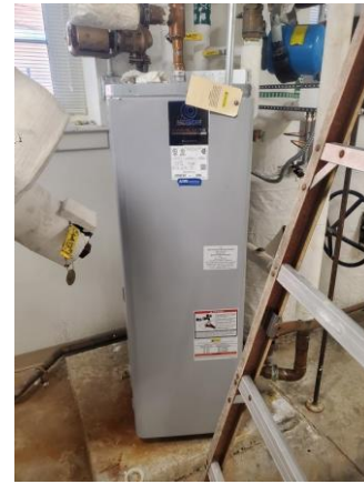
002070e 1/9/2023 Electric water heater Room 187
