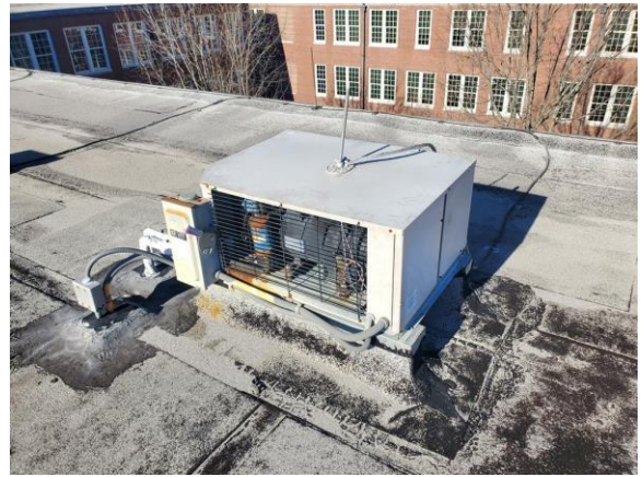
002023e 1/9/2023 Cold room refrigeration unit Roof
