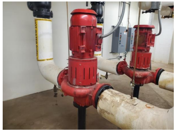
002057e 1/9/2023 Heating water pumps HWP-1 and 2 Room 153
