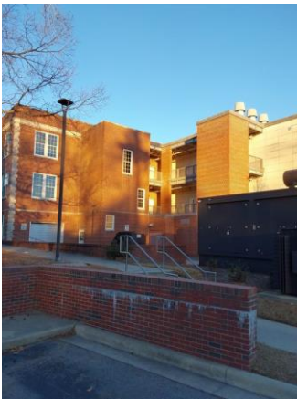
002104a 1/9/2023 Exterior balconies and brick efflorescence Southwest elevation
