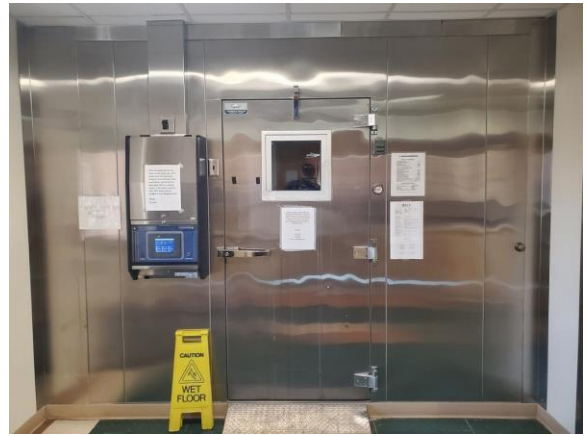
002049e 1/9/2023 Walk-in freezer Room 3224
