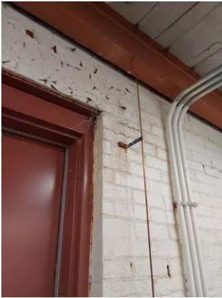
002016a 1/9/2023 Signs of water infiltration from exterior Roof attic
