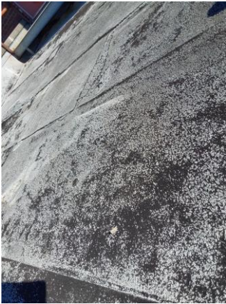
002002a 1/9/2023 Modified bitumen roof with blistering Roof
