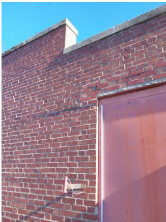
002015a 1/9/2023 Exterior brick damage on west end of attic Roof
