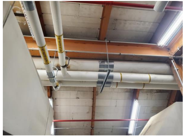
002014e 1/9/2023 Heating water supply and return pipe Room 450
