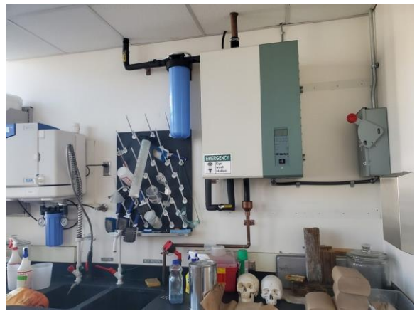
002048e 1/9/2023 Electric humidification device Room 3212
