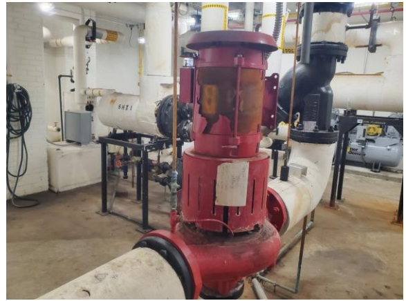
002058e 1/9/2023 Deteriorating paint on HWP-1 Room 153
