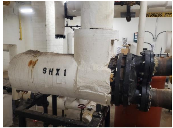
002064e 1/9/2023 Heating water shell-and-tube heat exchanger Room 153
