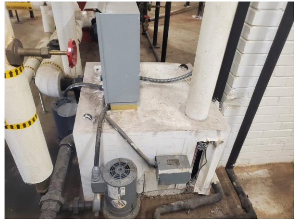
002061e 1/9/2023 Duplex condensate return system CU-1 Room 153
