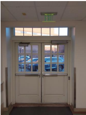
002110a 1/9/2023 Exit doors with power door operator East elevation
