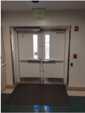
002062a 1/9/2023 Panic hardware with power door opener Room 3202
