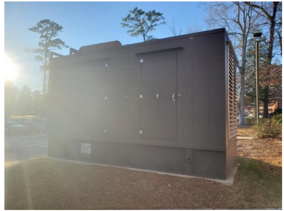
002076e 1/9/2023 450-kW diesel fire emergency generator Site
