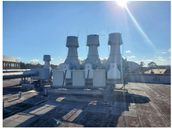
002002e 1/9/2023 Strobic exhaust fans AEF-1, LEF-1 through LEF-3 Roof
