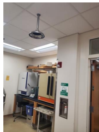
002040e 1/9/2023 Combination eyewash/safety shower Room 382
