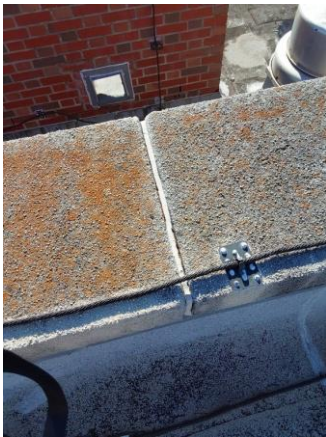
002009a 1/9/2023 Worn sealant on parapet joints Roof
