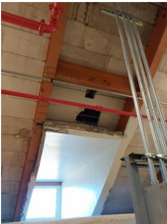
002012a 1/9/2023 Hole in substructure of terracotta roof Roof attic
