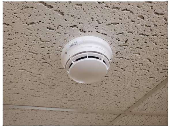
009006e 1/10/2023 Updated smoke/heat detector Third floor corridor
