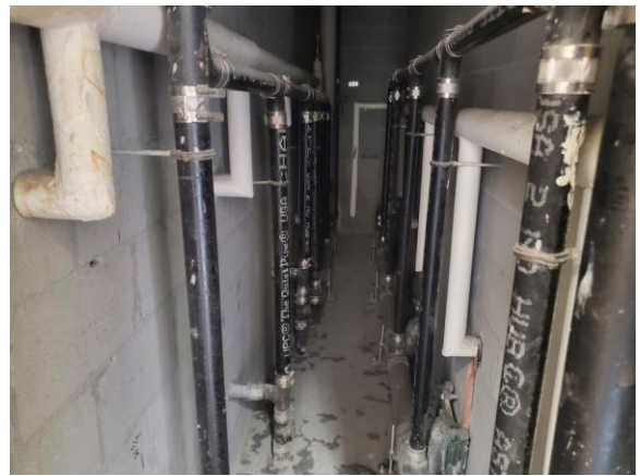
009036e 1/10/2023 Circa 2006 supply and waste piping First floor pipe chase
