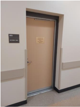
009058a 1/10/2023 Music room with sealed threshold and frame Room OB113
