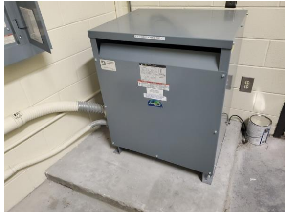
009040e 1/10/2023 Circa 2006 dry type transformer Electric B134
