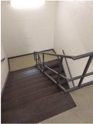
009013a 1/10/2023 Stair tower railing with noncompliant guardrail Southeast stair tower
