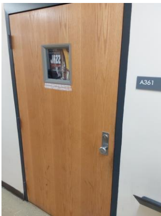
009012a 1/10/2023 Typical office door with knob hardware Room OA361
