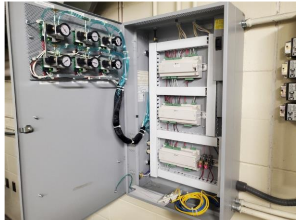
009029e 1/10/2023 Updated hardware and panelboard for HVAC controls Mechanical B135
