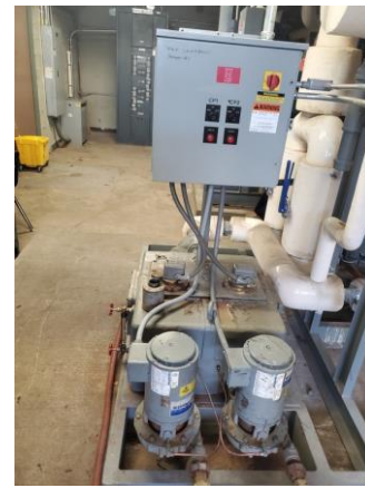
009056e 1/10/2023 Duplex condensate return system Mechanical 124
