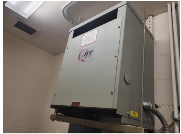
009001e 1/10/2023 Original dry-type transformer Room A380
