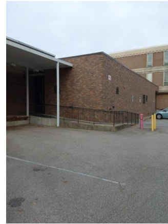
009121a 1/10/2023 Wheelchair ramp with noncompliant handrail East elevation
