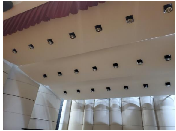
009038e 1/10/2023 Overview of stage lighting Stage 107A
