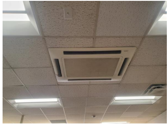
009070e 1/10/2023 Split system cassette Library 110
