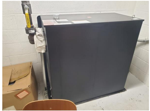
009044e 1/10/2023 Hydraulic elevator machine Elevator A126
