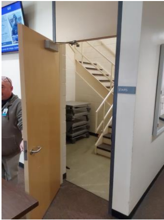
009067a 1/10/2023 Stair tower with noncompliant hardware Room 100A
