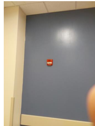
009095a 1/10/2023 Typical fire alarm for newer edition Room 101
