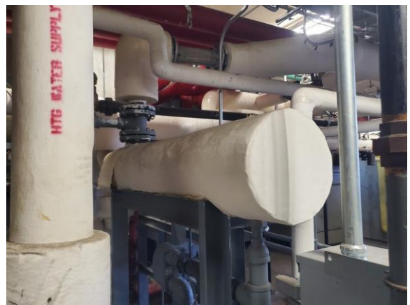
009057e 1/10/2023 Heating water shell-and-tube heat exchanger Mechanical 124
