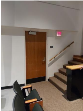
009090a 1/10/2023 Exit door with noncompliant hardware Room OC107
