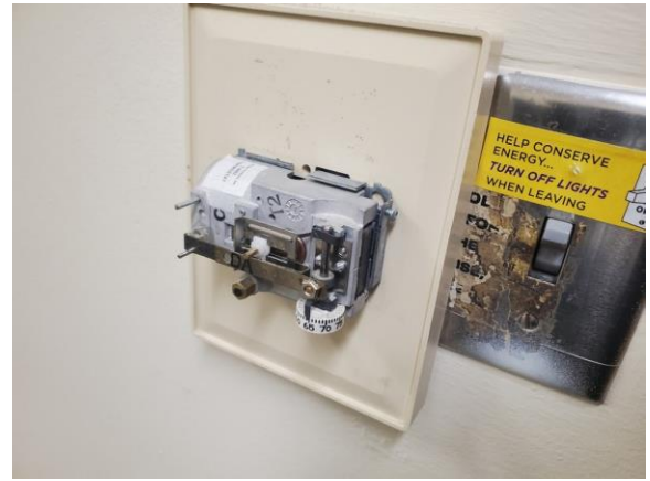
009013e 1/10/2023 Aged electromechanical thermostat to be updated Third floor corridor
