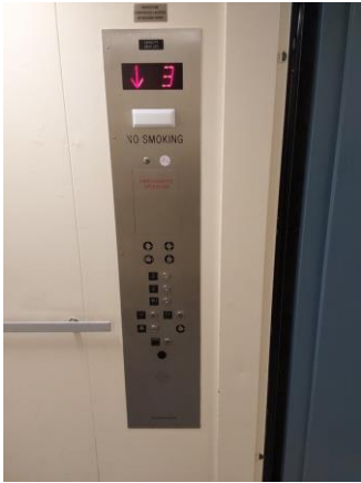
009001a 1/10/2023 Freight elevator panel Room OA399
