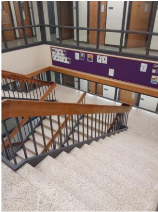
009016a 1/10/2023 Noncompliant stair railing with missing handrail Central stair
