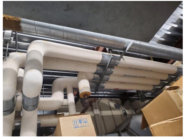
009022e 1/10/2023 Circa 2006 chilled and heating water piping Mechanical B135
