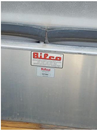
009071a 1/10/2023 Roof hatch nameplate West roof
