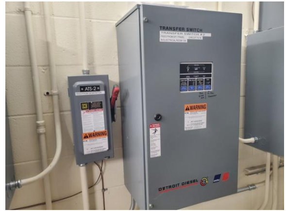
009019e 1/10/2023 Automatic transfer switch 2 Mechanical B135
