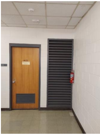
009038a 1/10/2023 Mechanical louver Room 101
