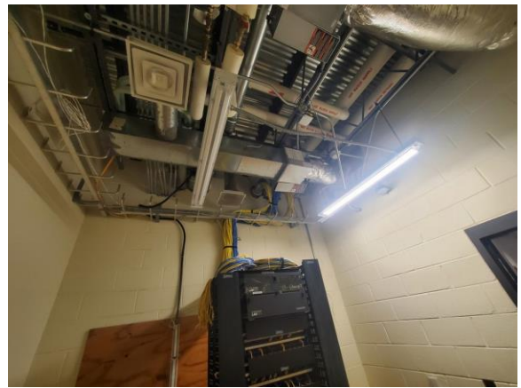
009039e 1/10/2023 Server rack that needs drip pan installed above Data B112
