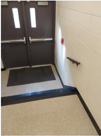
009047a 1/10/2023 Noncompliant stair railing Room 114
