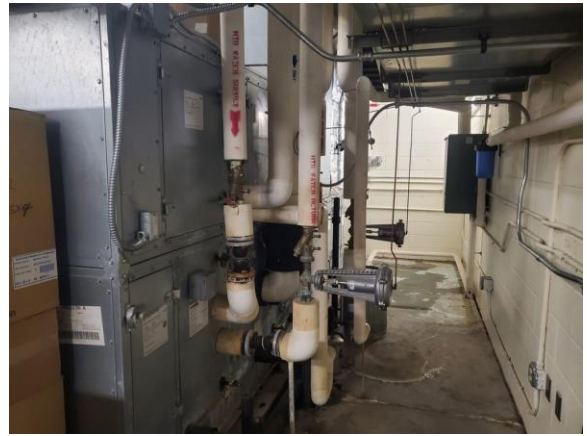
009025e 1/10/2023 Air handler unit AHU-5 Mechanical B135
