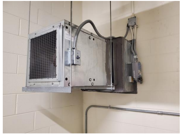
009043e 1/10/2023 Through-wall exhaust fan Fire Pump room B132
