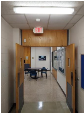
009039a 1/10/2023 Noncompliant exit doors with safety glass Room 101
