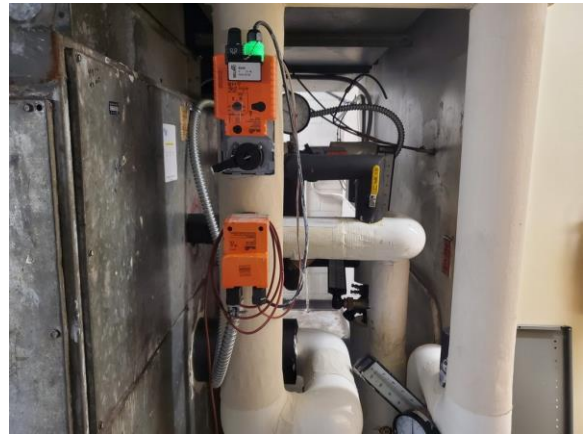
009034e 1/10/2023 Updated electronic Belimo actuating damper Mechanical C208
