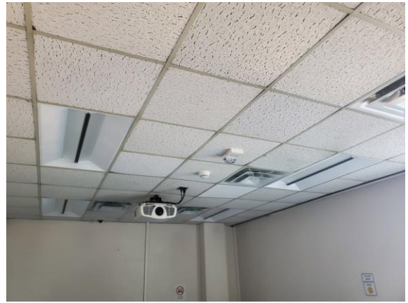
009010e 1/10/2023 Overview of classroom and office lighting Room A300
