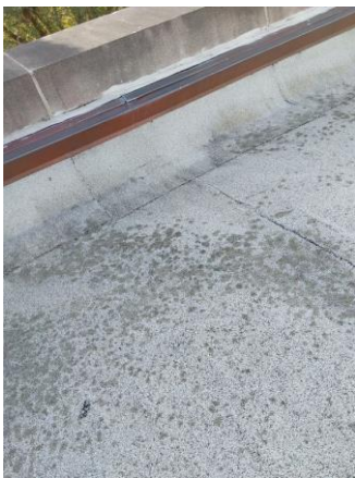
009072a 1/10/2023 Blister on newer portion of roof West roof
