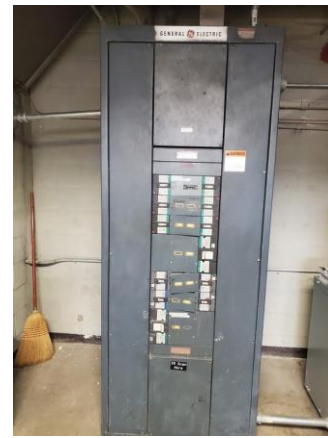
009065e 1/10/2023 Original electrical system main switchboard Mechanical 124
