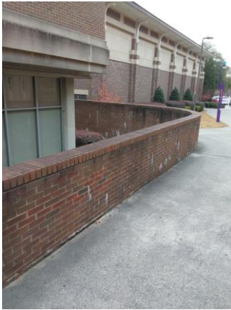
009104a 1/10/2023 Efflorescence on brick retaining wall West elevation
