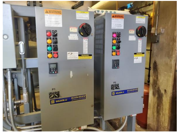
009059e 1/10/2023 HW pump variable speed drives Mechanical 124
