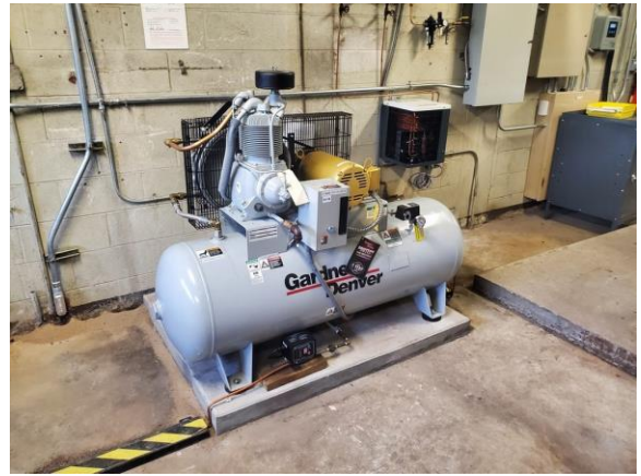
009055e 1/10/2023 Reciprocating air compressor and dryer for control system Mechanical 124
