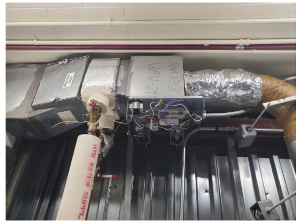
009015e 1/10/2023 VAV terminal assembly Mechanical B135
