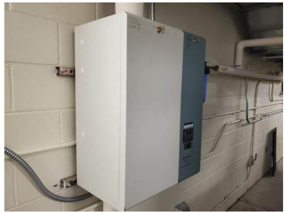
009027e 1/10/2023 Electric humidification for AHU-5 Mechanical B135
