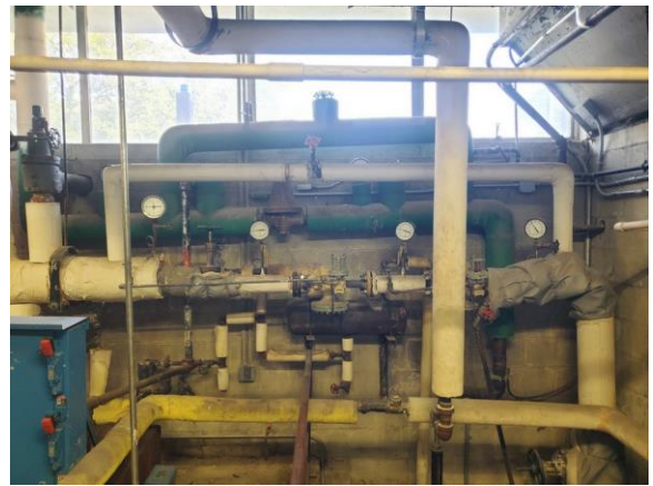
009048e 1/10/2023 Steam pressure reducing station and relief valve Mechanical 124
