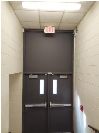
009048a 1/10/2023 Exit door showing panic hardware Room 114
