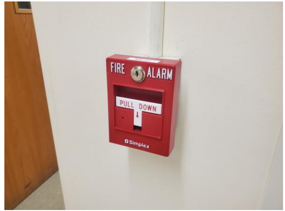
009008e 1/10/2023 Updated manual fire alarm pull station Third floor corridor
