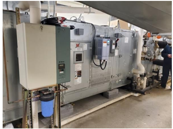
009031e 1/10/2023 Variable speed AHU-4 and electric humidifier Mechanical B201
