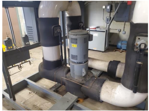
009064e 1/10/2023 Chilled water system pump Mechanical 124
