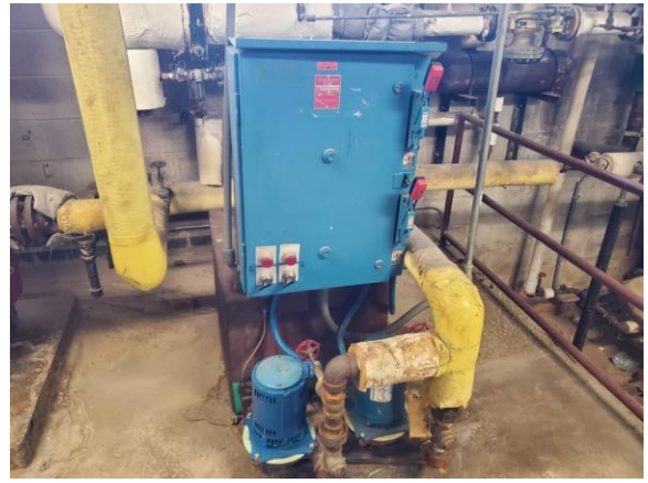
009049e 1/10/2023 Duplex condensate return system Mechanical 124
