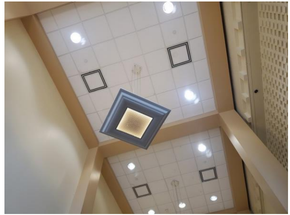
009035e 1/10/2023 Decorative and recessed lighting Lobby B101
