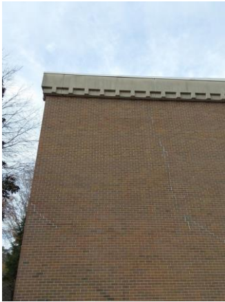
009120a 1/10/2023 Cracks from settling on exterior wall East elevation
