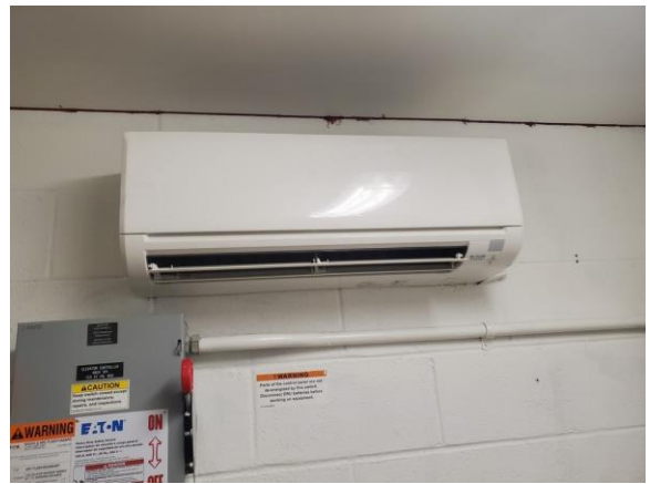
009045e 1/10/2023 Split system blower assembly Elevator A126
