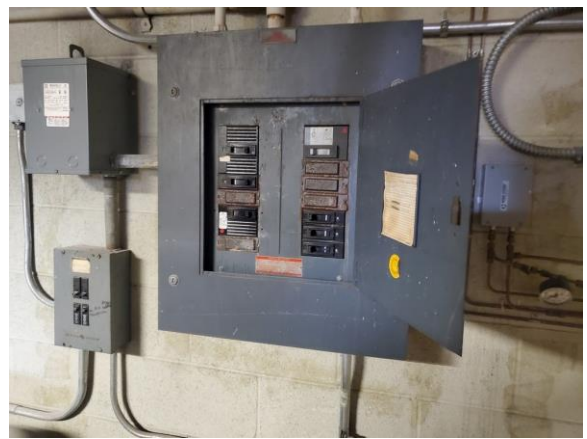
009066e 1/10/2023 Aged secondary electric panelboard Mechanical 124
