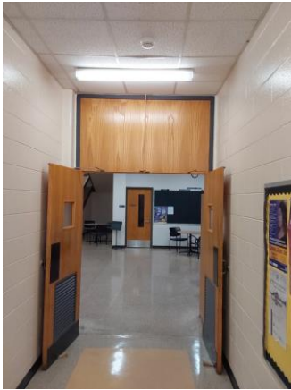
009043a 1/10/2023 Corridor exit doors without safety glass Room 101
