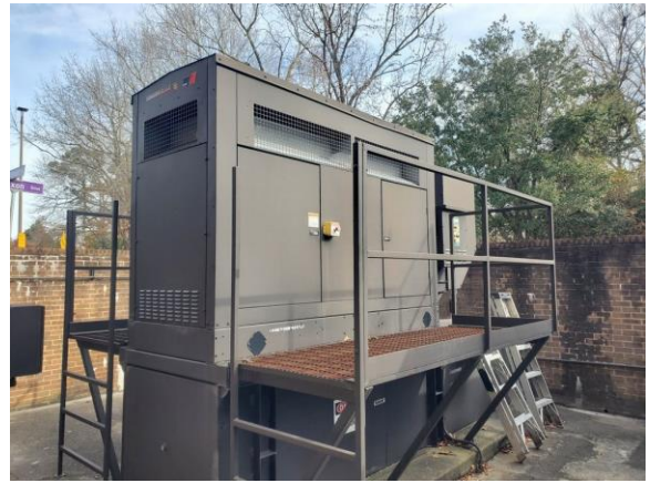
009068e 1/10/2023 Emergency generator Exterior
