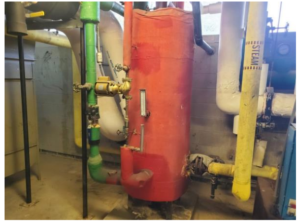
009050e 1/10/2023 Aged steam to water domestic water heater and pump Mechanical 124
