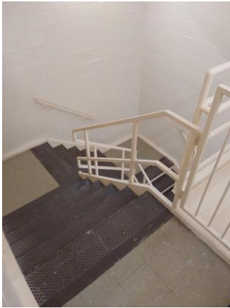
009068a 1/10/2023 Noncompliant stair handrail Room 100A
