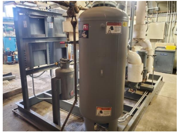
009061e 1/10/2023 Heating water expansion tank Mechanical 124
