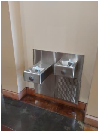
009063a 1/10/2023 Dual height water fountains Room OB101
