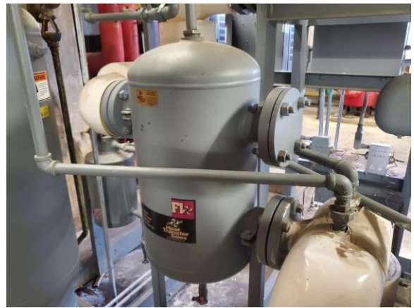
009060e 1/10/2023 Heating water air separator Mechanical 124
