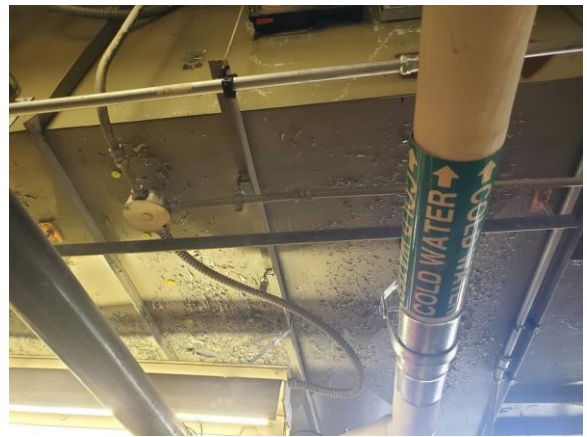
009054e 1/10/2023 Flaking paint on HVAC system ductwork Mechanical 124
