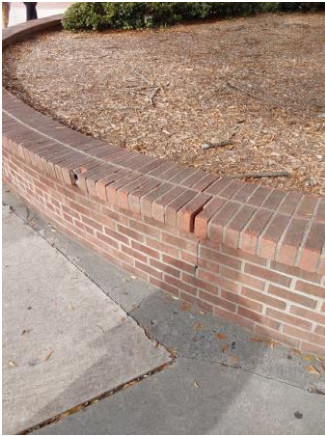
009114a 1/10/2023 Brick landscaping wall damaged South elevation
