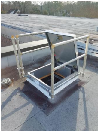
009070a 1/10/2023 Roof hatch with fiberglass fault protection West roof
