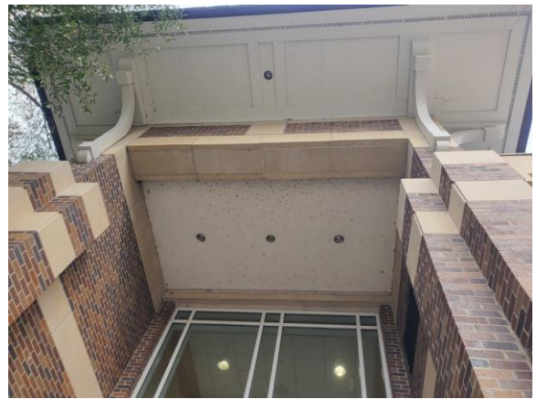
009078e 1/10/2023 Recessed can style lighting Exterior
