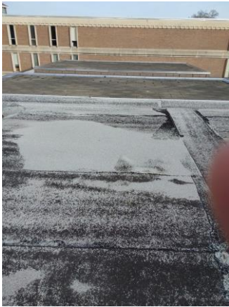
009074a 1/10/2023 Roof blister on older portion of roof South roof
