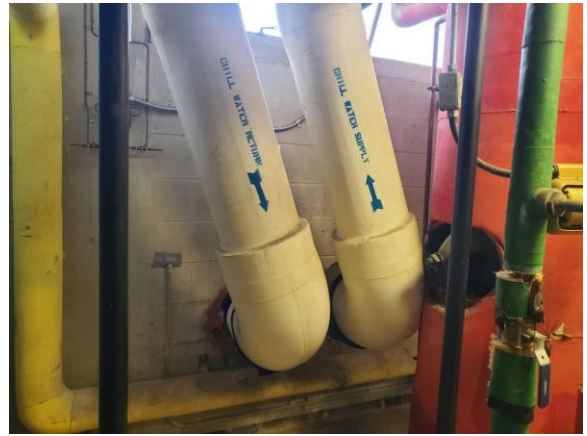
009046e 1/10/2023 Main chilled water from utility system Mechanical 124
