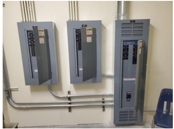
009041e 1/10/2023 Circa 2006 electrical panelboards Electric B134
