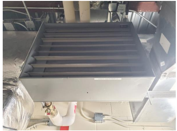
009026e 1/10/2023 Hydronic unit heater Mechanical B135
