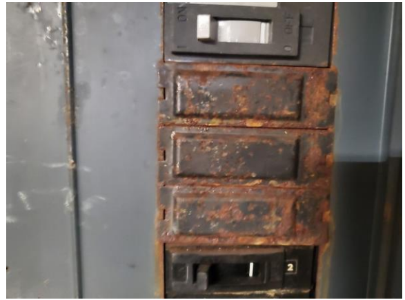
009067e 1/10/2023 Corroded spacer covers in original panelboard Mechanical 124
