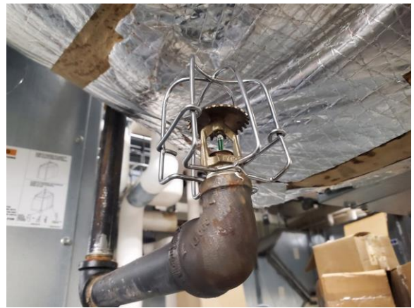
009024e 1/10/2023 Fire suppression system sprinkler head for 2006 addition Mechanical B135
