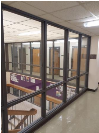
009015a 1/10/2023 Safety glass adjacent to corridor Central stair
