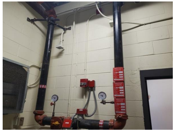
009042e 1/10/2023 Fire suppression system riser for 2006 addition Fire Pump room B132
