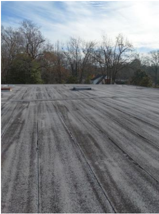
009076a 1/10/2023 Missing fall protection South roof
