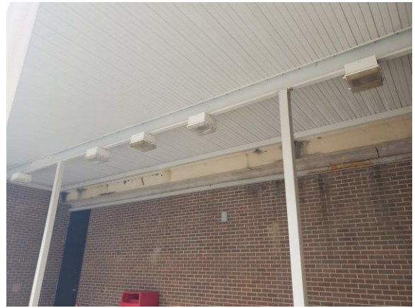
009077e 1/10/2023 Surface mounted HID light fixtures Loading dock
