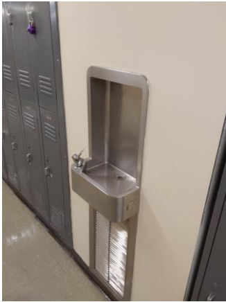
009031a 1/10/2023 Typical water fountain North corridor
