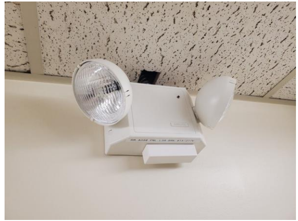
009007e 1/10/2023 Updated emergency light fixture Third floor corridor
