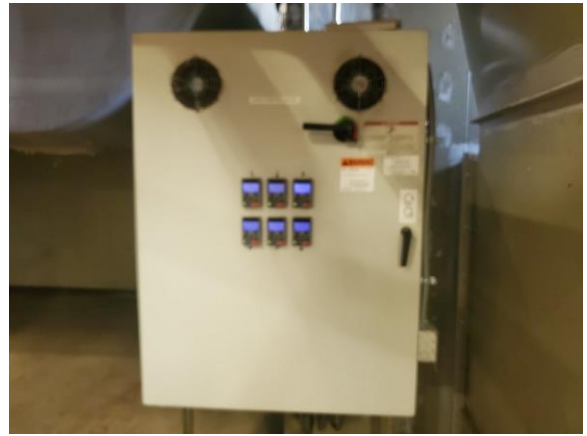
009052e 1/10/2023 VFDs for AHU-2 fan wall system Mechanical 124
