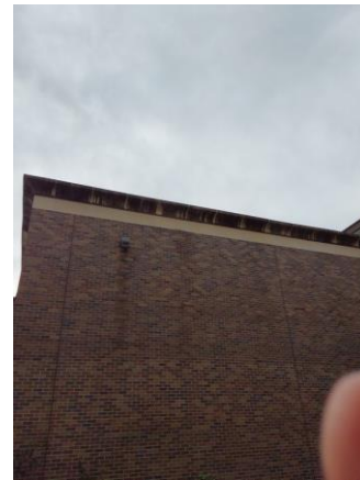
009107a 1/10/2023 Dirty roof eave West elevation
