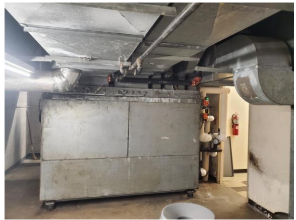
009033e 1/10/2023 Dual duct air handler AHU-3 Mechanical C208
