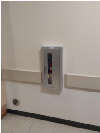
009061a 1/10/2023 Typical fire extinguisher cabinet Room OB117
