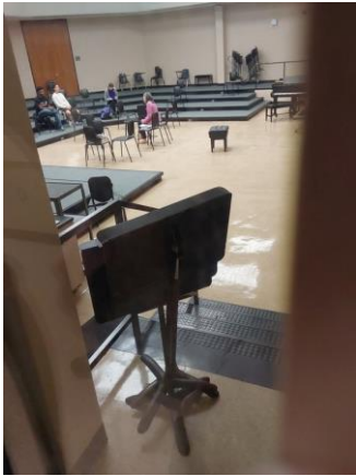
009096a 1/10/2023 Classroom stair with noncompliant handrails Room OB136
