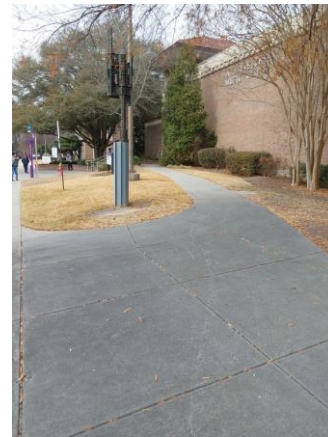
009119a 1/10/2023 ADA ramp needs landing South elevation
