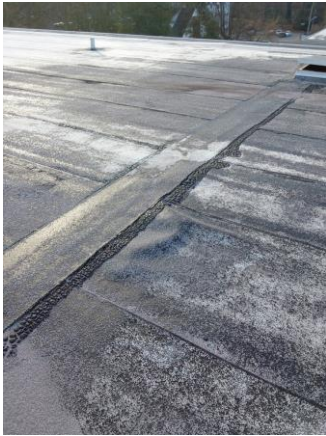
009002a 1/10/2023 Roof blistering Roof
