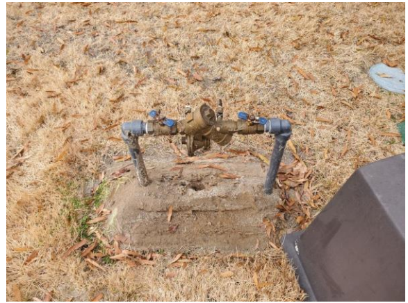
009079e 1/10/2023 Irrigation system backflow Site
