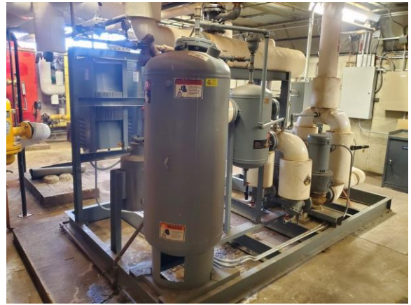
009062e 1/10/2023 Overview of heating water system skid Mechanical 124
