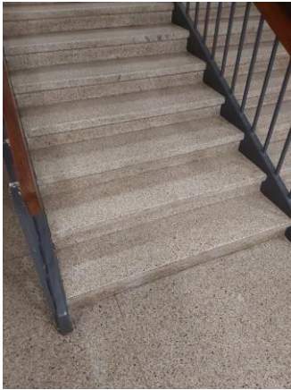
009040a 1/10/2023 Central stair without tread finish Room 101
