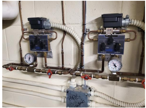
009028e 1/10/2023 Hybrid HVAC controls Mechanical B135
