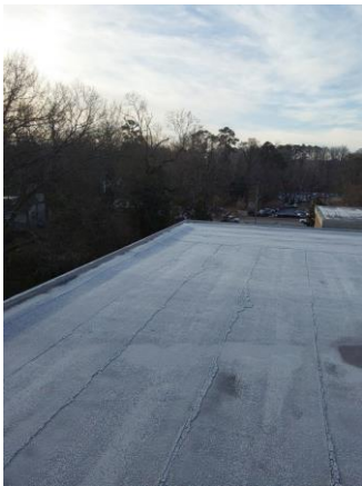
009003a 1/10/2023 Lack of fall protection on roof perimeter Roof
