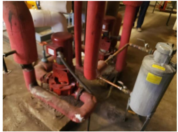
009053e 1/10/2023 Heating water supply pumps Mechanical 124
