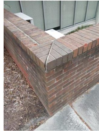
009105a 1/10/2023 Damaged brick on retaining wall West elevation
