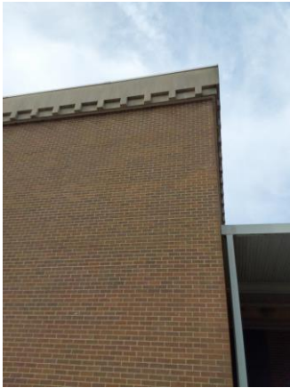
009122a 1/10/2023 Crack on exterior east wall East elevation
