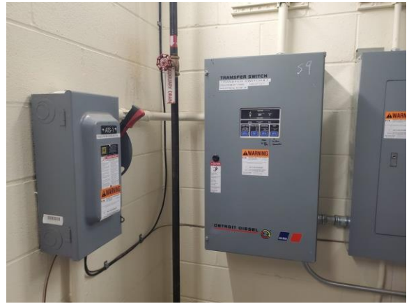
009017e 1/10/2023 Automatic transfer switch 1 Mechanical B135
