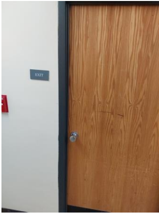
009014a 1/10/2023 Stair tower with noncompliant exit door Southeast stair tower
