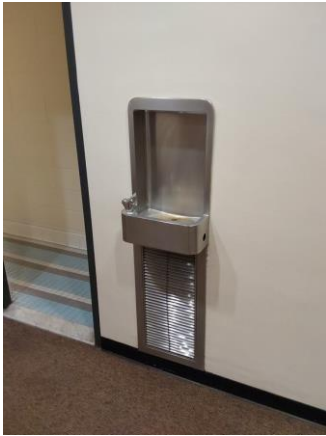
009064a 1/10/2023 Noncompliant inset water fountain Room OB101
