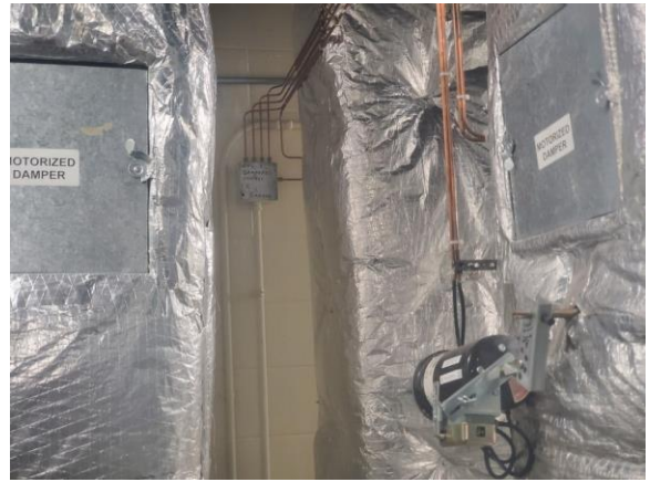
009023e 1/10/2023 Compressed air pipe for pneumatic operation Mechanical B135
