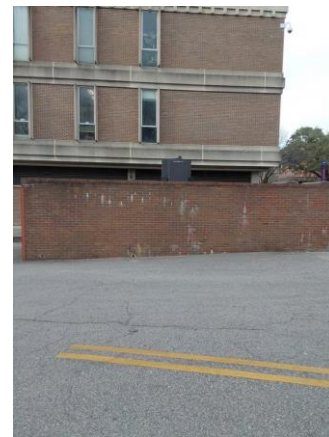
009101a 1/10/2023 Efflorescence on brick East elevation
