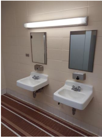
009011a 1/10/2023 Noncompliant wall-hung lavatories Room OA381
