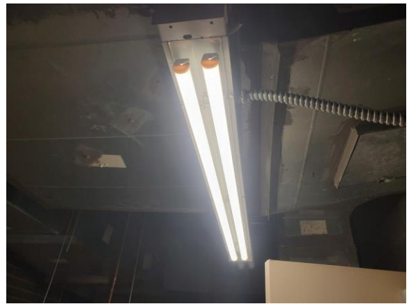
009030e 1/10/2023 Surfaced mounted lighting with T12 lamps Mechanical B201
