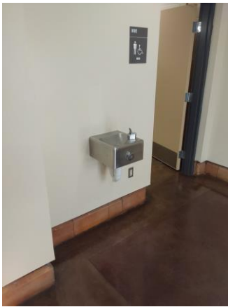
009065a 1/10/2023 Noncompliant water fountain Room OB101
