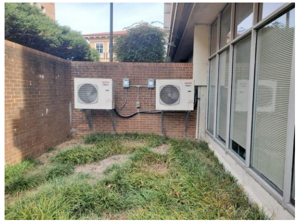
009071e 1/10/2023 Split system air-cooled condensers for library Exterior
