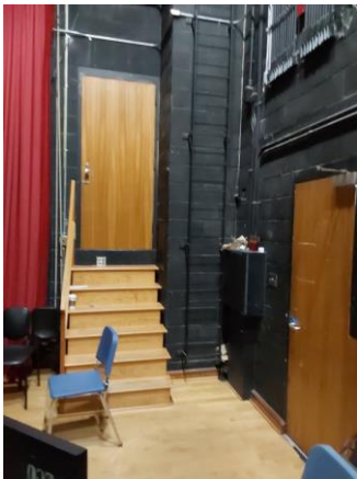
009088a 1/10/2023 Backstage stairs with noncompliant railing Room OC107
