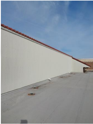
009073a 1/10/2023 Painted corrugated metal on newer roof edition West roof
