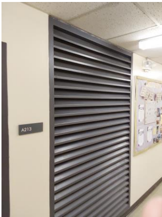
009030a 1/10/2023 Mechanical louver Second floor, room OA213
