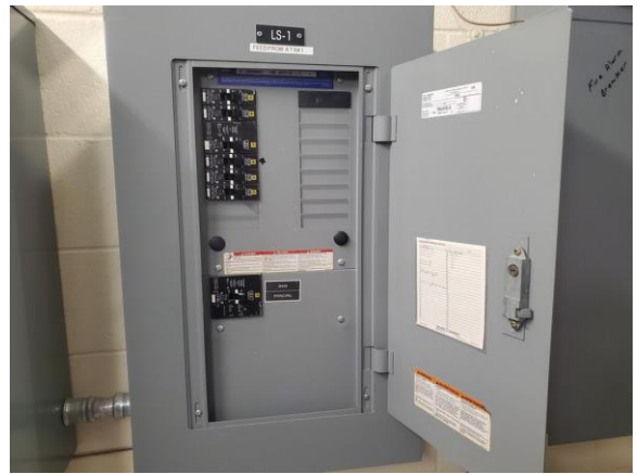
009018e 1/10/2023 Circa 2006 electrical panelboard Mechanical B135
