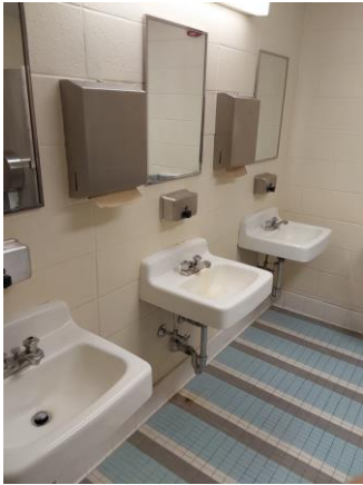
009080a 1/10/2023 Noncompliant lavatories Room OC109
