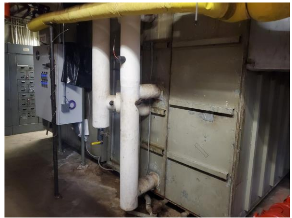
009063e 1/10/2023 Air handler AHU-1 with updated fan wall Mechanical 124
