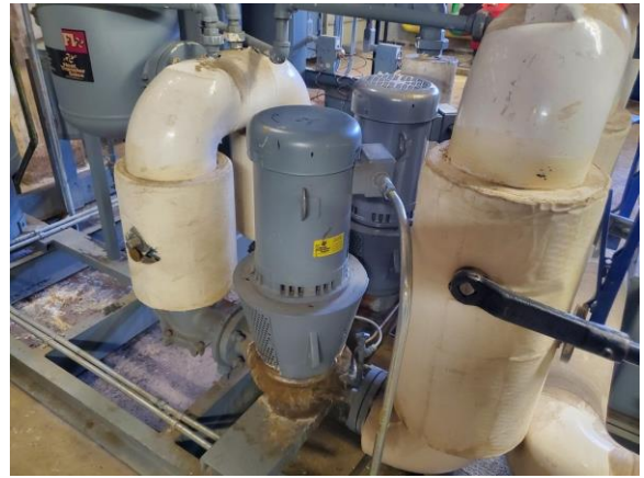
009058e 1/10/2023 Heating water supply pumps Mechanical 124
