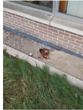
009103a 1/10/2023 Hole along north elevation grade North elevation
