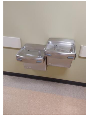
009099a 1/10/2023 Dual height water fountains Room OB123
