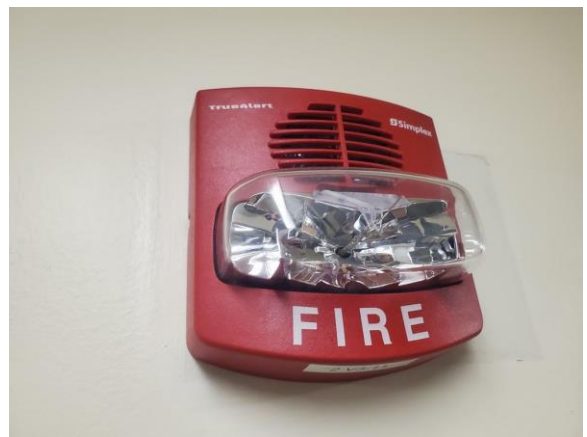
009012e 1/10/2023 Updated fire alarm notifier Third floor corridor
