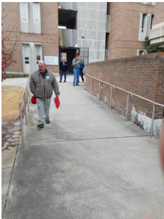
009106a 1/10/2023 Wheelchair ramp with noncompliant handrails West elevation
