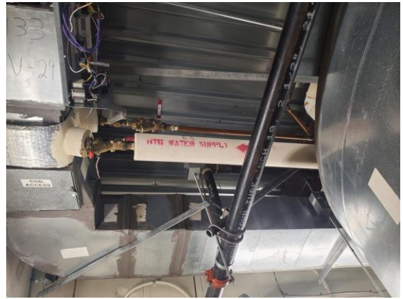
009016e 1/10/2023 Heating water supply pipe and metal ductwork Mechanical B135
