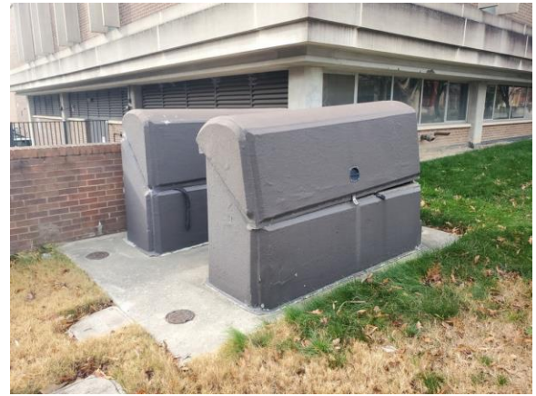
009074e 1/10/2023 Main backflow preventer housing Site
