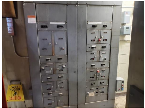
009069e 1/10/2023 Aged motor control center Mechanical 124
