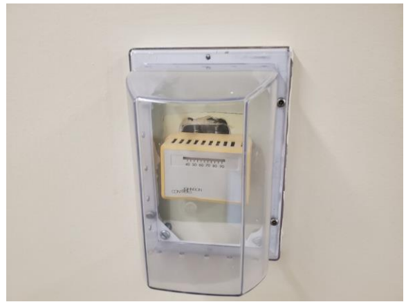
009009e 1/10/2023 Original thermostat to be replaced Third floor corridor
