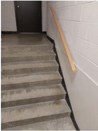
009092a 1/10/2023 Noncompliant handrails Loading area
