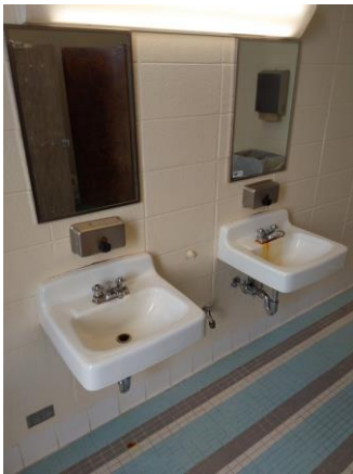
009027a 1/10/2023 Noncompliant lavatories Room OA370B
