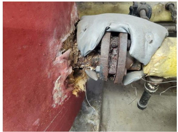
009051e 1/10/2023 Moderate corrosion on domestic water heater Mechanical 124
