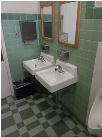
001A068a 1/12/2023 Wall-hung lavatories and ceramic floor and wall finishes Room 108a
