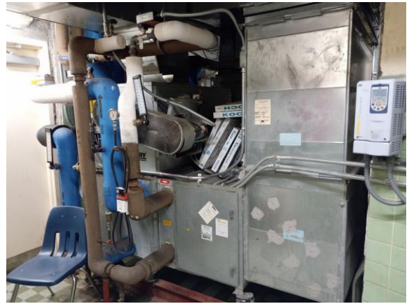
001A037e 1/12/2023 Circa 1997 air handler AHU-20 Mechanical 203
