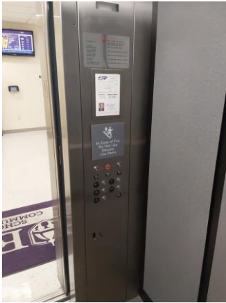
001A052a 1/12/2023 Elevator control panel Elevator 4
