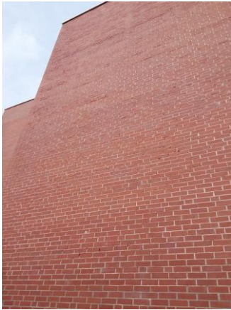
001A010a 1/12/2023 Brick deterioration on south facing wall South elevation
