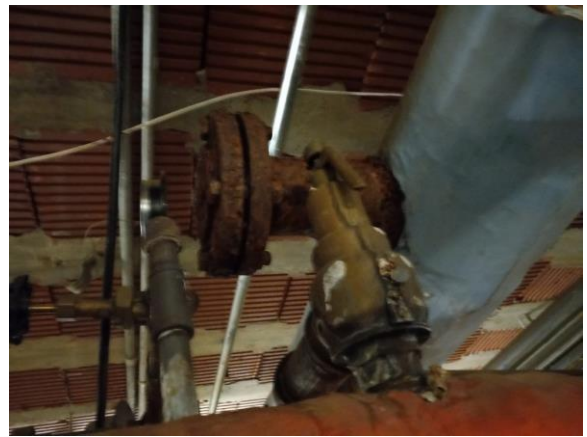
001A021e 1/12/2023 Steam safety relief valve Room B01
