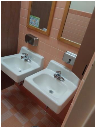
001A070a 1/12/2023 Wall-hung lavatories Room 108B
