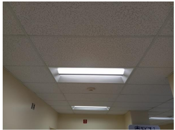
001A033e 1/12/2023 2x4 recessed lighting with LED retrofit Second floor corridor
