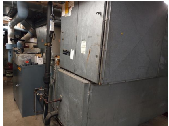
001A009e 1/12/2023 Air handler AHU-14 Room B01
