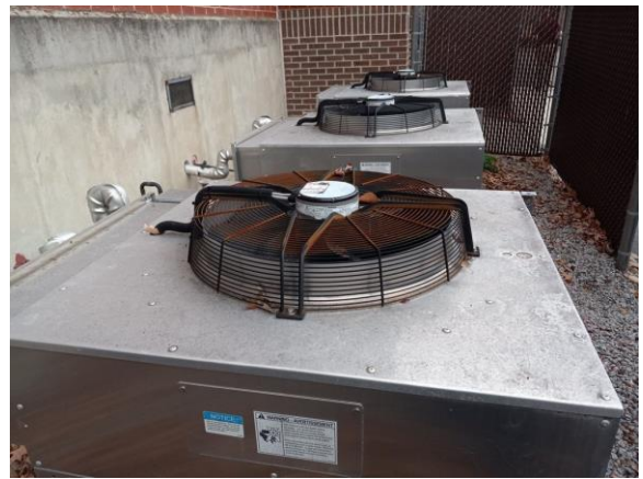
001A054e 1/12/2023 Computer room air cooled condensers Exterior
