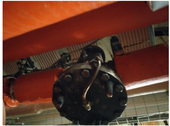
001A020e 1/12/2023 Pressure reducing valve Room B01
