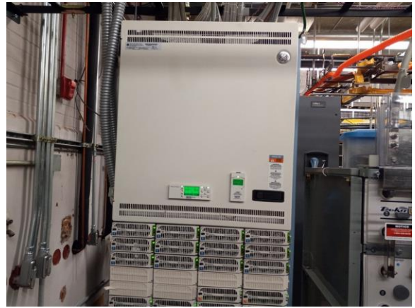
001A031e 1/12/2023 Network emergency power battery inverter Room B01A
