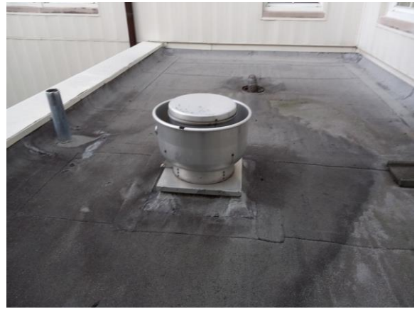
001A029e 1/12/2023 Rooftop exhaust fan Lower roof
