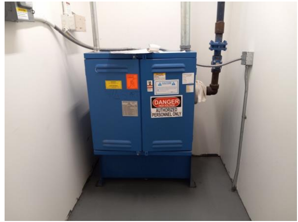
001A046e 1/12/2023 Hydraulic elevator machine Elevator 099
