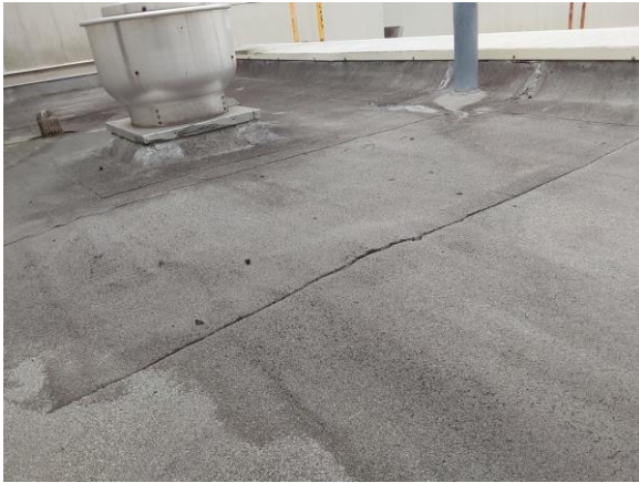
001A023a 1/12/2023 Roof blister Roof
