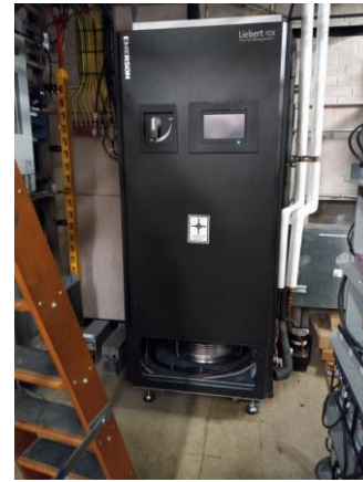
001A022e 1/12/2023 Computer room AC unit 5 Room B01A
