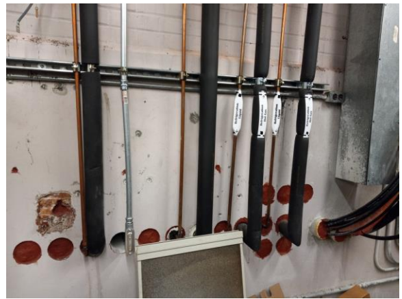
001A027e 1/12/2023 Various piping systems Room B01A
