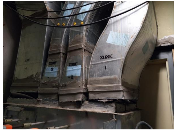
001A040e 1/12/2023 Zoned, metal HVAC ductwork Mechanical 203B
