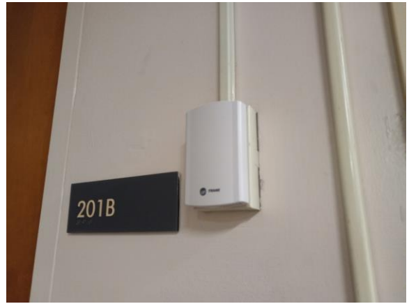
001A044e 1/12/2023 Updated Trane sensor and temperature controller Room 201
