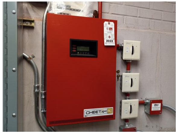
001A024e 1/12/2023 HFC 227 fire suppression system controller Room B01A
