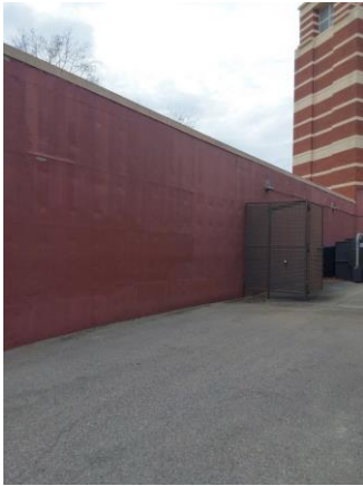
001A019a 1/12/2023 Back of south mechanical wall South wall
