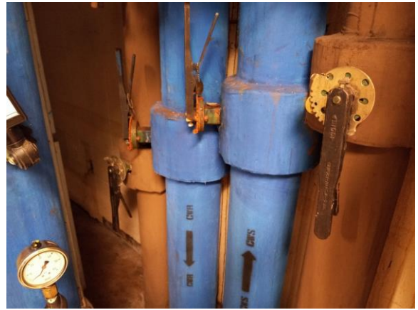
001A043e 1/12/2023 Chilled and heating water distribution pipe Mechanical 297
