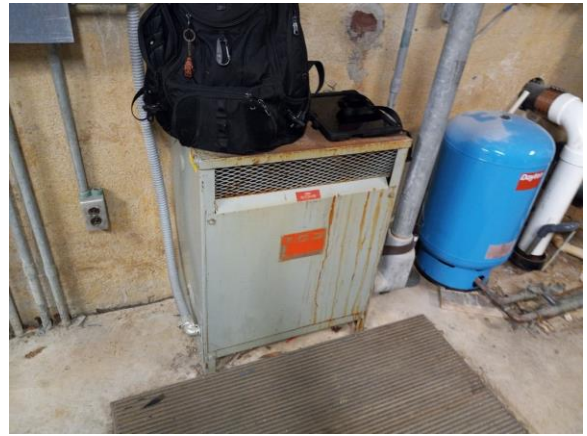
001A002e 1/12/2023 Circa 1990 dry-type transformer Room B01
