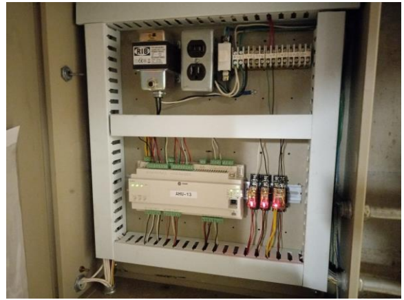
001A013e 1/12/2023 Modernized controls Room B01
