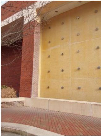
001A002a 1/12/2023 Water stains on wall West elevation
