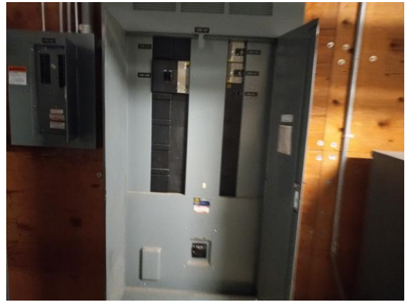
001A007e 1/12/2023 600-amp panelboard LPB5 Room B01
