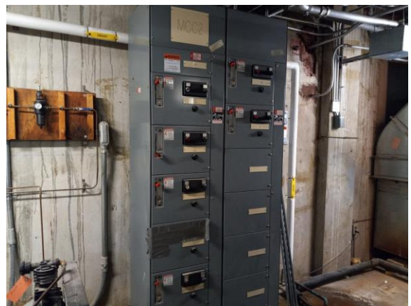
001A006e 1/12/2023 Motor control center MCC-2 Room B01
