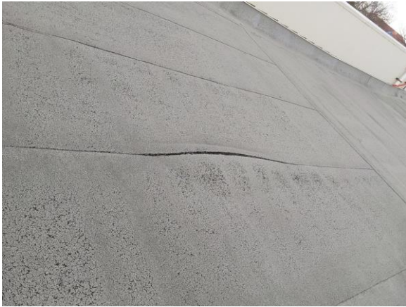
001A026a 1/12/2023 Roof blister Roof
