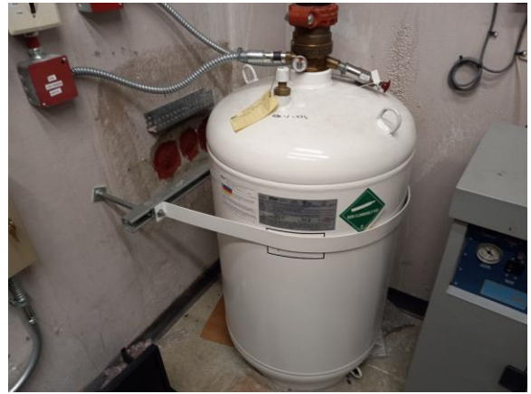
001A025e 1/12/2023 HFC 227 fire suppression system chemical storage tank Room B01A
