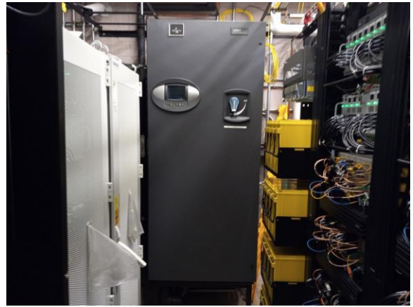
001A023e 1/12/2023 Computer room AC unit CRU-1 Room B01A
