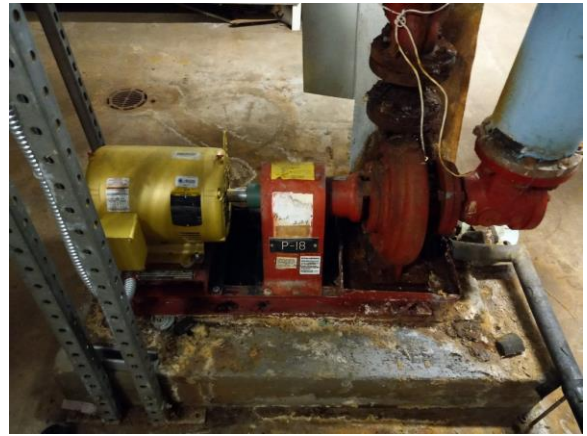
001A019e 1/12/2023 Chilled water pump P-18 Room B01
