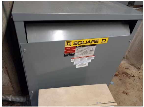
001A001e 1/12/2023 150-kVA dry-type transformer TDAS1 Room B01
