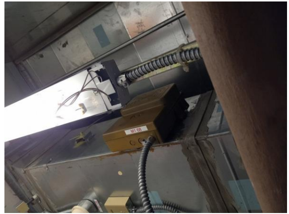
001A038e 1/12/2023 Lighting showing retrofit kit Mechanical 203
