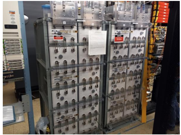
001A026e 1/12/2023 Network emergency power battery bank Room B01A
