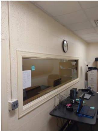
001A043a 1/12/2023 Wall with possible asbestos Room 205B
