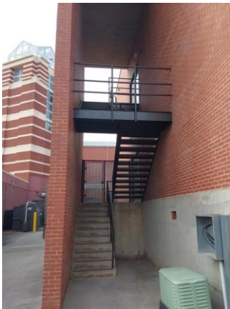
001A009a 1/12/2023 Exterior fire stair without handrail South elevation
