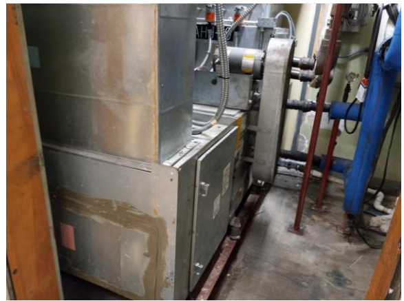
001A039e 1/12/2023 Circa 1997 air handler AHU-19 Mechanical 203B
