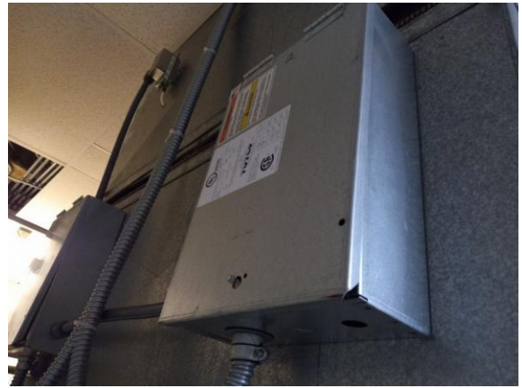
001A049e 1/12/2023 Electric duct heater Mechanical 104
