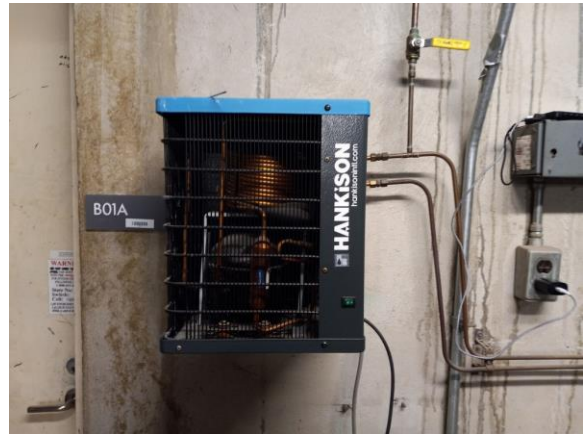
001A004e 1/12/2023 Refrigerated air dryer Room B01
