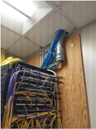
001A055a 1/12/2023 Missing fire blocking in conduit Room 102D
