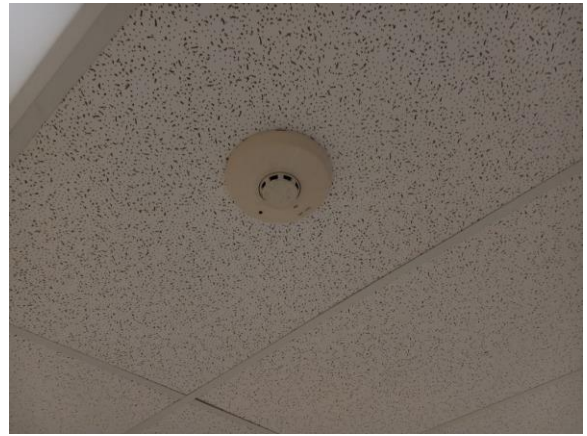
001A034e 1/12/2023 Fire alarm system detector Second floor corridor
