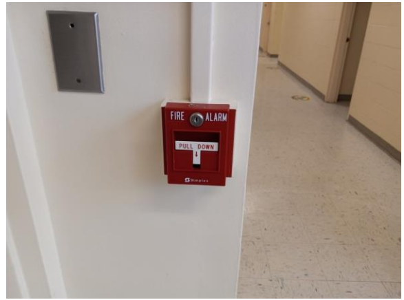
001A041e 1/12/2023 Fire alarm system pull station Second floor corridor
