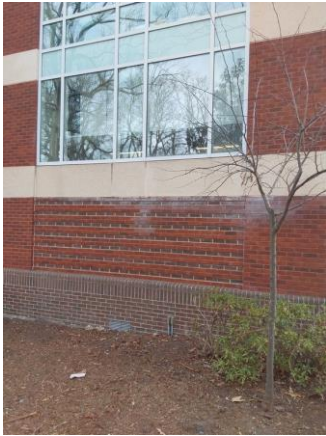
001A004a 1/12/2023 Brick efflorescence North elevation
