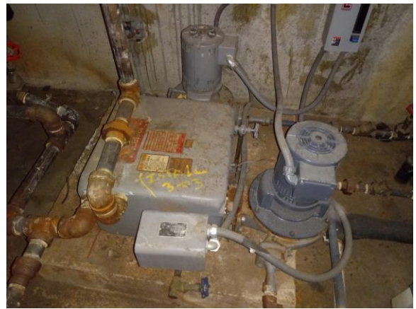
001A015e 1/12/2023 Duplex condensate return unit Room B01
