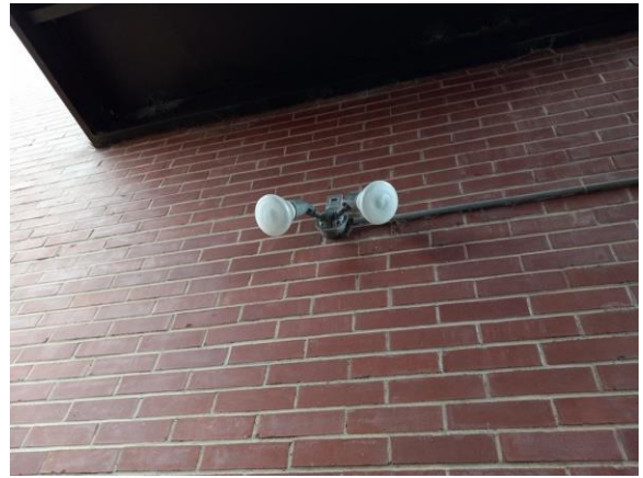
001A053e 1/12/2023 Aged flood light Exterior
