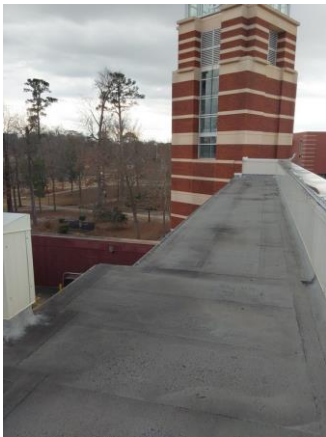
001A027a 1/12/2023 Fall protection needed over water wall Roof
