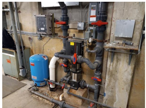
001A003e 1/12/2023 Water wall feature pump skid Room B01
