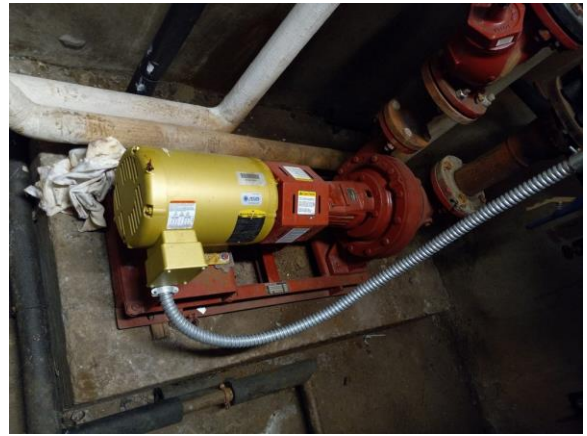
001A017e 1/12/2023 Heating water pump Room B01
