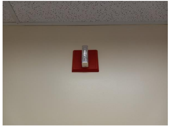
001A035e 1/12/2023 Fire alarm system notifier Second floor corridor
