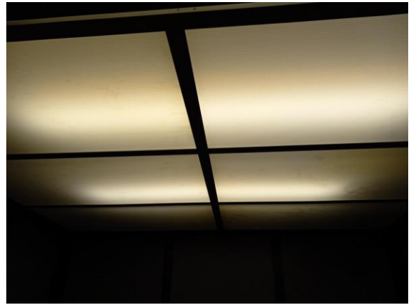
001A032e 1/12/2023 Elevator lighting Elevator
