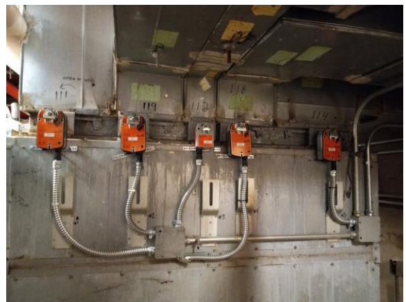
001A018e 1/12/2023 Updated controls on air handler AHU-16 Room B01
