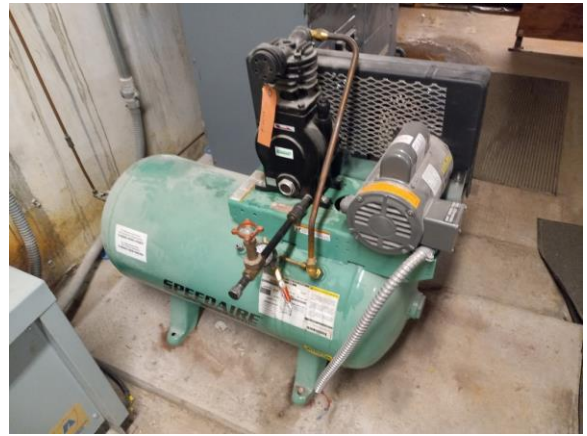
001A005e 1/12/2023 Air compressor Room B01
