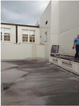
001A031a 1/12/2023 Grime on metal siding Roof
