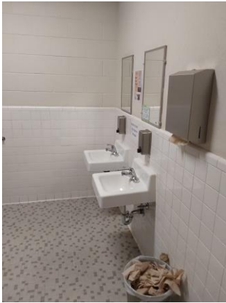
001A072a 1/12/2023 Wall-hung lavatories Room 109B
