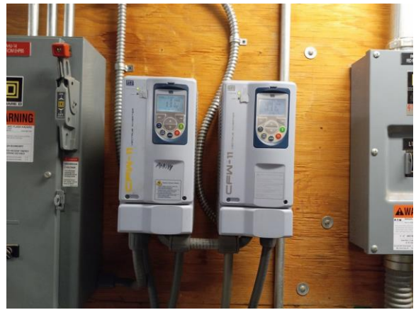
001A011e 1/12/2023 Variable speed drives for AHU-13 and AHU-14 Room B01
