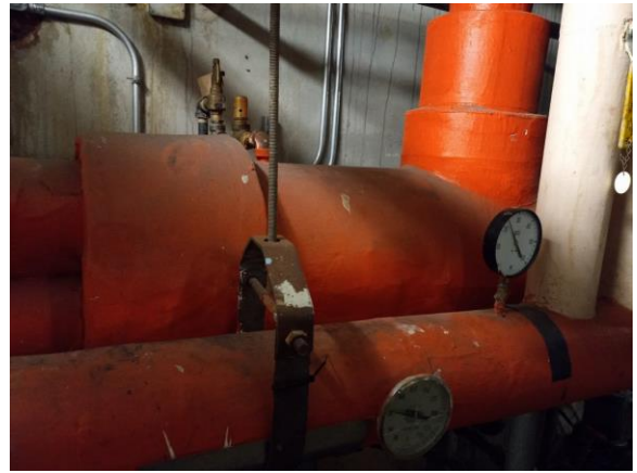
001A016e 1/12/2023 Shell and tube heat exchanger Room B01
