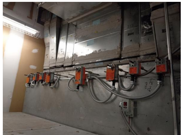
001A042e 1/12/2023 Modernized electronic actuators Mechanical 297
