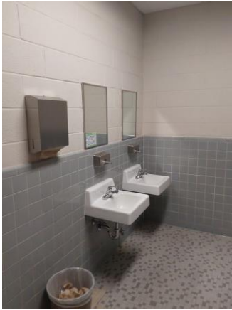
001A062a 1/12/2023 Ceramic floor and wall tile, painted upper wall, and wall-hung lavatories Room 109a
