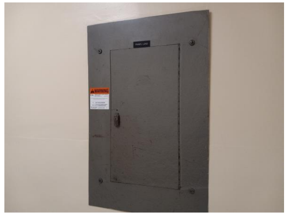
001A036e 1/12/2023 Aged secondary electric system panelboard Second floor corridor
