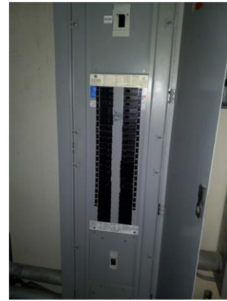
001A050e 1/12/2023 Circa 1994 electrical panelboard Mechanical 104
