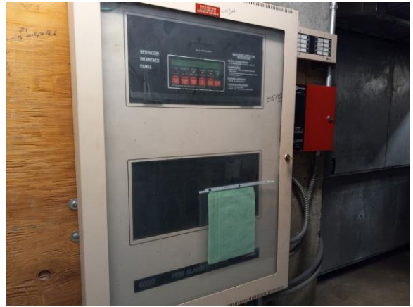
001A008e 1/12/2023 Fire alarm control panel Room B01
