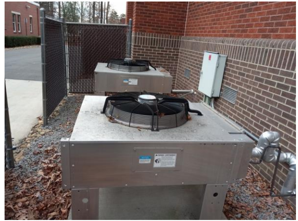
001A055e 1/12/2023 Computer room air-cooled condensers Site
