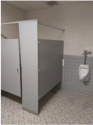
001A061a 1/12/2023 Urinal, toilet partition and ceramic wall and floor finishes Room 109a
