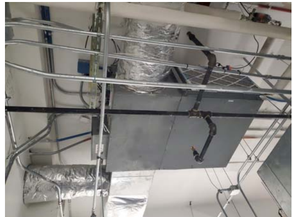
001051e 1/12/2023 Variable volume terminal unit with modernized controls Mechanical 2911
