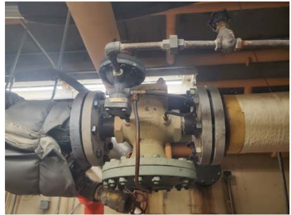
001077e 1/12/2023 Steam pressure reducing valve Mechanical B909
