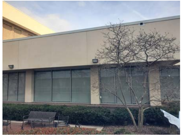
001064e 1/12/2023 Surface mounted HID lighting Interior courtyard
