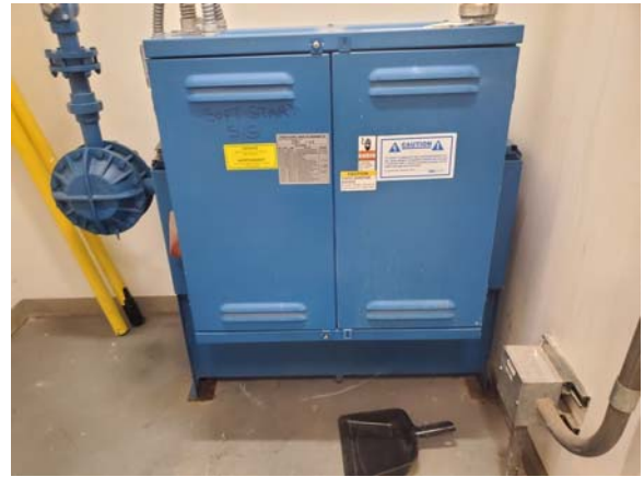
001062e 1/12/2023 Hydraulic elevator machine Elevator Machine 1910
