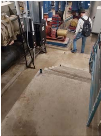
001124a 1/12/2023 Mechanical room railing has been cut Room B021
