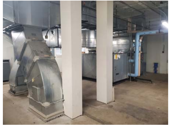
001049e 1/12/2023 Overview of mechanical room and equipment Mechanical 2911
