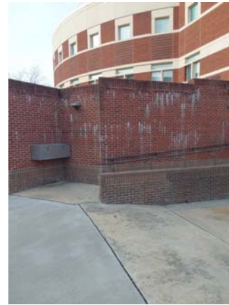
001144a 1/12/2023 Brick efflorescence South elevation
