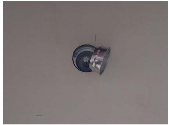
001124e 1/12/2023 Damaged, recessed light fixture Exterior
