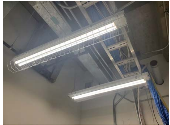
001008e 1/12/2023 Pendant style lighting for mechanical, electrical, data, etc. Data 4901
