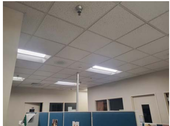
001018e 1/12/2023 Typical 2x4 lighting for offices, work spaces, and stacks Workroom 4002
