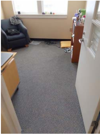
001064a 1/12/2023 Worn carpet and office areas Room 2600
