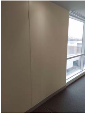
001049a 1/12/2023 Wall crack at structural joint Room 3085
