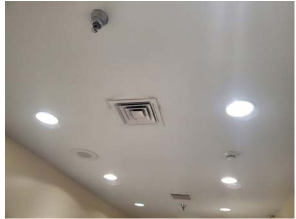
001013e 1/12/2023 Recessed lighting and sprinkler head Corridor 4008
