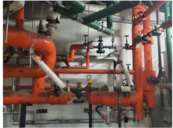
001097e 1/12/2023 Central steam station Mechanical B901
