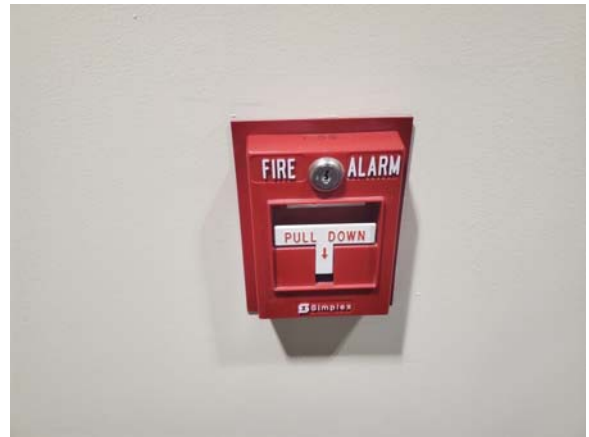
001015e 1/12/2023 Fire alarm pull station Corridor 4008
