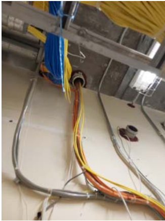
001118a 1/12/2023 Data room missing fire blocking Room B907
