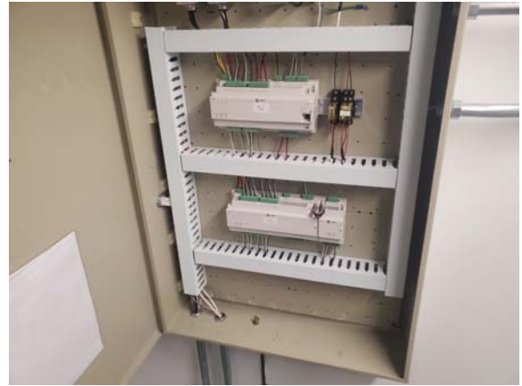
001007e 1/12/2023 Modernized HVAC system controllers and software Mechanical 4903
