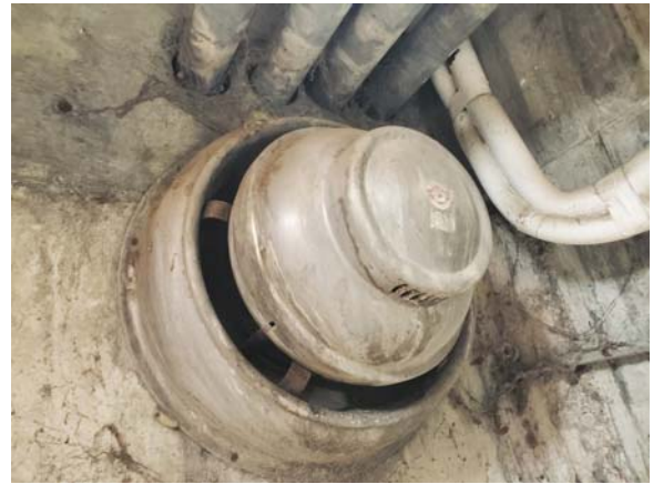
001071e 1/12/2023 Aged through wall exhaust fan Mechanical B909
