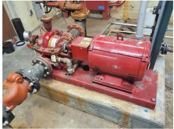
001073e 1/12/2023 Electric fire pump Mechanical B909
