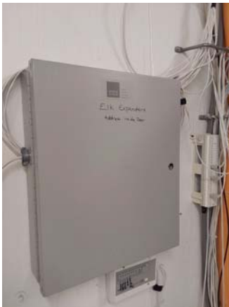
001033a 1/12/2023 Fire protection access control box Room 3907
