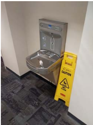
001069a 1/12/2023 Single height water fountain Room 2039
