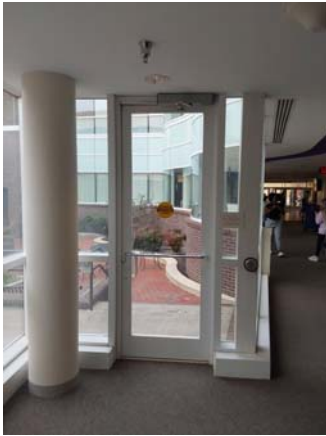
001109a 1/12/2023 Exit door with power door operator Room 1104
