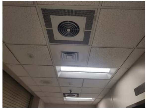
001056e 1/12/2023 Ceiling mounted electric unit heaters Corridor 1060
