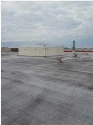
001004a 1/12/2023 Rotunda roof with missing fall protection Rotunda roof
