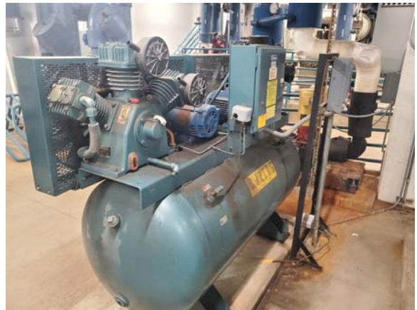
001108e 1/12/2023 Multi-stage HVAC control system air compressor Mechanical B901
