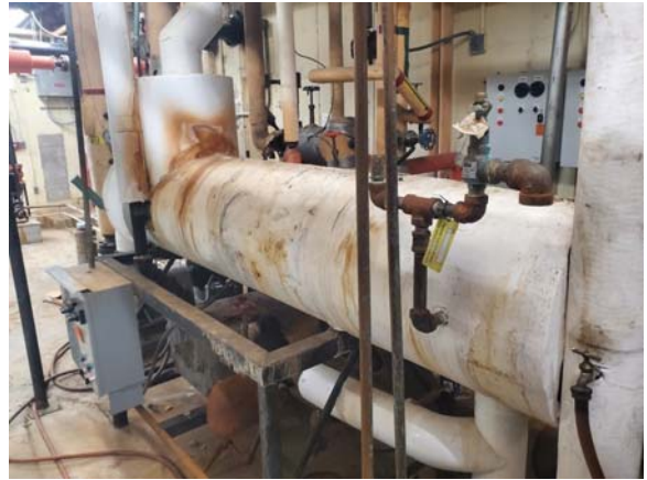
001079e 1/12/2023 Circa 2012 steam-to-water heat exchanger Mechanical B909
