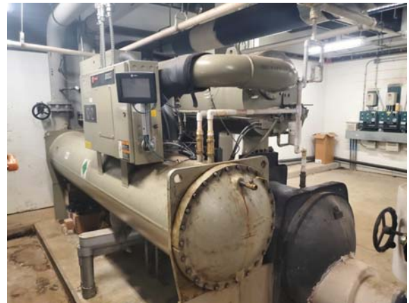
001111e 1/12/2023 Water cooled chiller C-2 Mechanical B901
