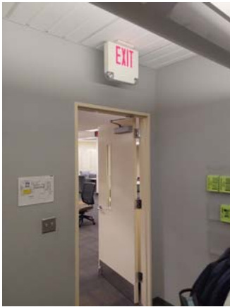
001119a 1/12/2023 Exit door without panic hardware Room B100
