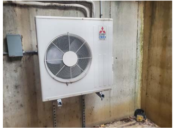
001070e 1/12/2023 Ductless split system condenser unit Mechanical B909
