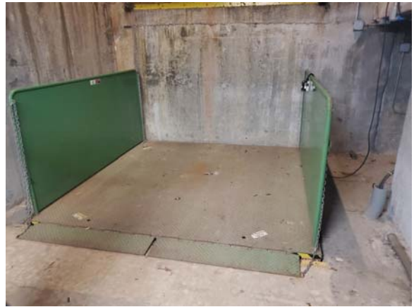
001116e 1/12/2023 Hydraulic lift Mechanical service tunnel
