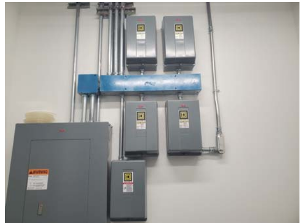
001012e 1/12/2023 Circa 1997 lighting contactors Electrical 4900
