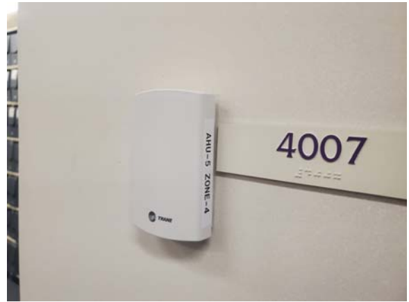
001020e 1/12/2023 Modernized HVAC system thermostat/controller Workroom 4002
