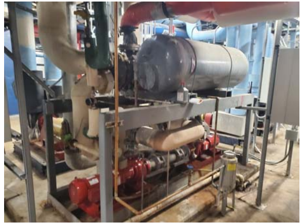
001107e 1/12/2023 Heating hot water skid with HEX, tanks, and pumps Mechanical B901
