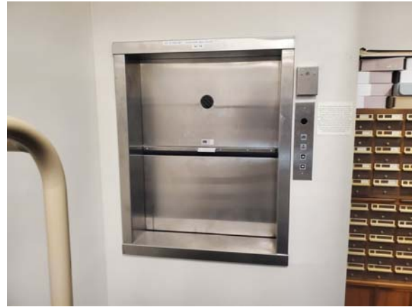
001019e 1/12/2023 Two-stop dumbwaiter Workroom 4002
