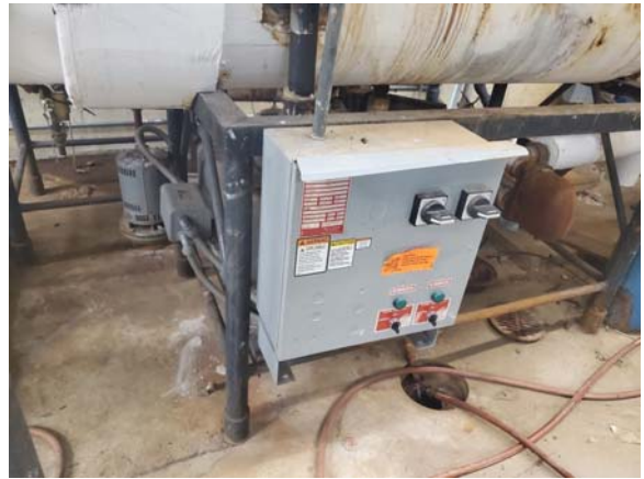
001080e 1/12/2023 Duplex condensate return unit Mechanical B909
