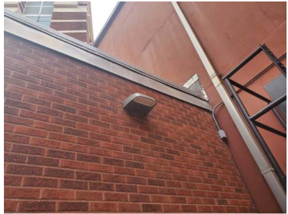
001122e 1/12/2023 Surface mounted LED light fixture Exterior
