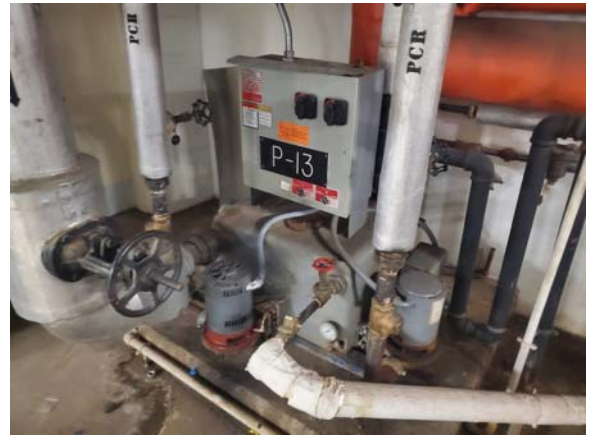
001098e 1/12/2023 Duplex condensate return system P-13 Mechanical B901
