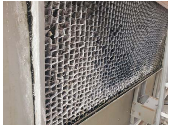
001119e 1/12/2023 Corroded and damaged tower fill Site
