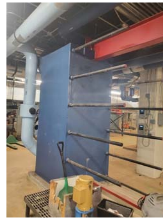
001090e 1/12/2023 Free cooling heat exchanger HE-1 Mechanical B901
