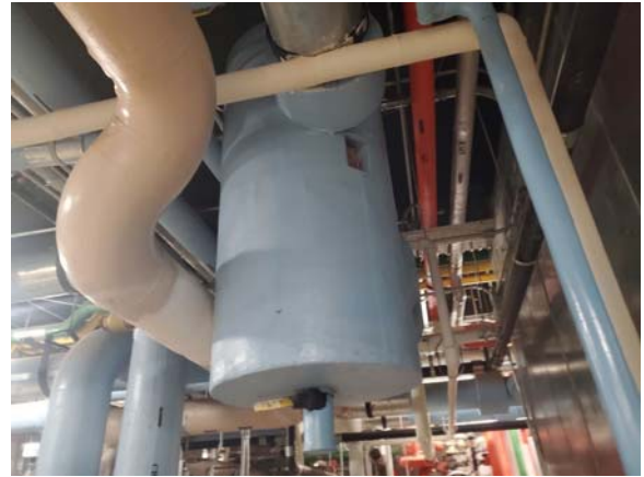
001091e 1/12/2023 Chilled water system air separator Mechanical B901
