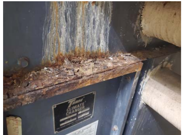
001045e 1/12/2023 Moderate corrosion on 1976 vintage air handler Mechanical 3900
