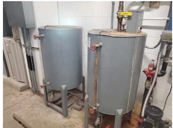
001102e 1/12/2023 Glycol mixing and storage equipment Mechanical B901
