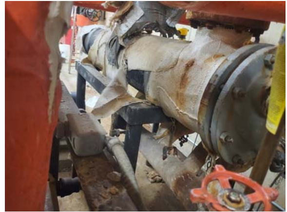
001082e 1/12/2023 Aged shell-and-tube heat exchanger Mechanical B909
