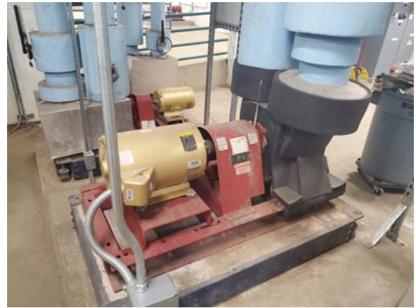
001104e 1/12/2023 Chilled water system pumps Mechanical B901
