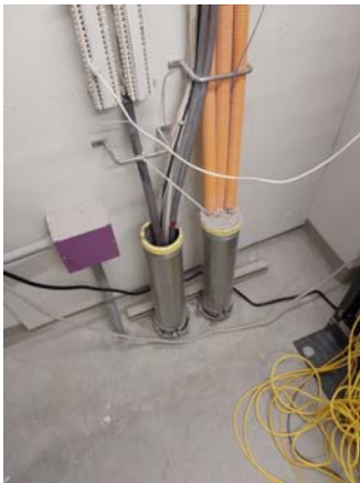
001060a 1/12/2023 Missing fire blocking Room 2906
