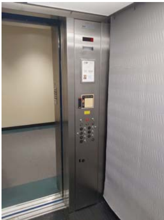
001015a 1/12/2023 Elevator control panel Elevator 2
