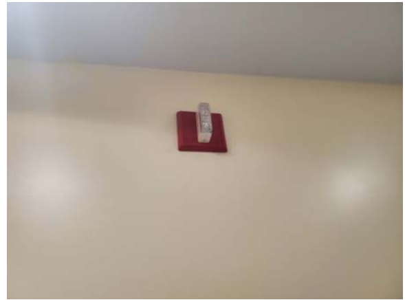
001014e 1/12/2023 Fire alarm system notifier circa 1997 Corridor 4008
