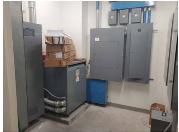
001023e 1/12/2023 Circa 1997 transformer and electrical panelboards Electrical 3905
