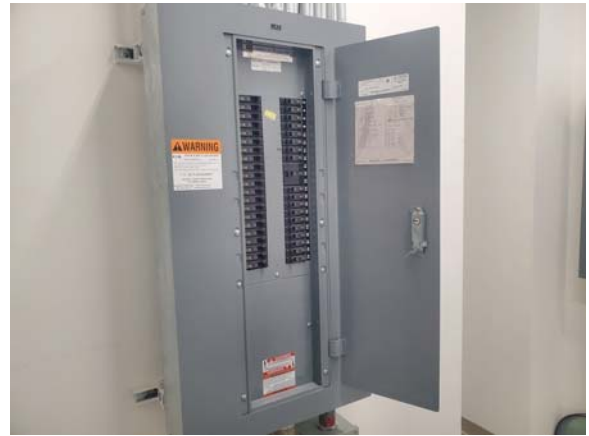
001011e 1/12/2023 Circa 1997 electrical panelboard Electrical 4900
