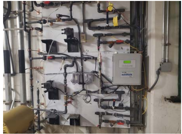
001101e 1/12/2023 Water treatment station Mechanical B901
