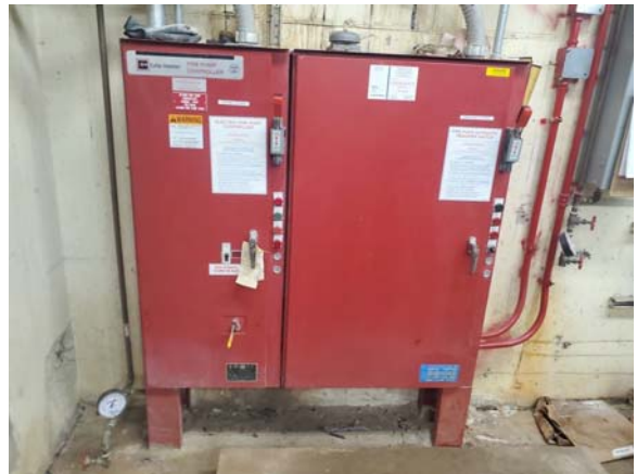
001075e 1/12/2023 Fire pump controller and transfer switch Mechanical B909
