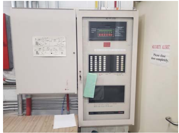
001113e 1/12/2023 Addressable fire alarm control panel Mechanical B901
