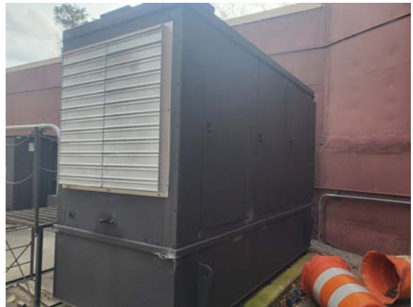
001117e 1/12/2023 400-kW diesel fire emergency generator Site
