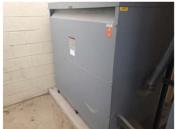
001072e 1/12/2023 225-kVA dry-type transformer Mechanical B909
