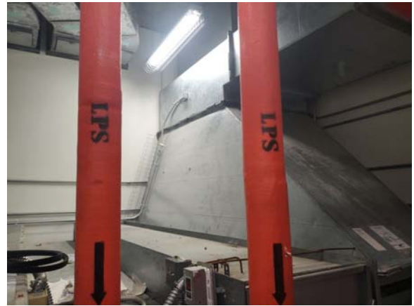
001035e 1/12/2023 Low pressure steam pipe for humidification Mechanical 3904
