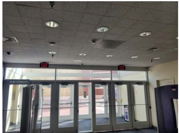
001066e 1/12/2023 Aged and recessed lobby lighting Lobby 1105
