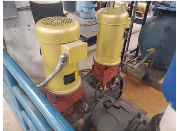
001109e 1/12/2023 Glycol system pumps with minor corrosion Mechanical B901
