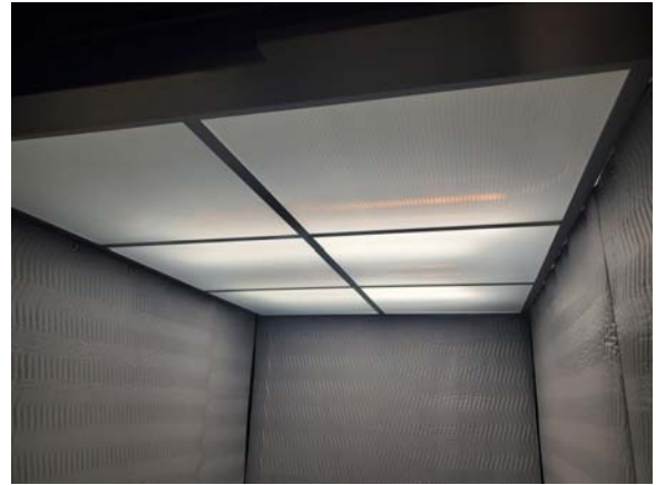
001022e 1/12/2023 Hydraulic elevator 2 lighting Elevator 2
