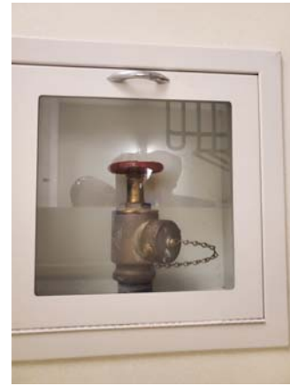
001016e 1/12/2023 Fire hose connection point Stair 1911S (10)
