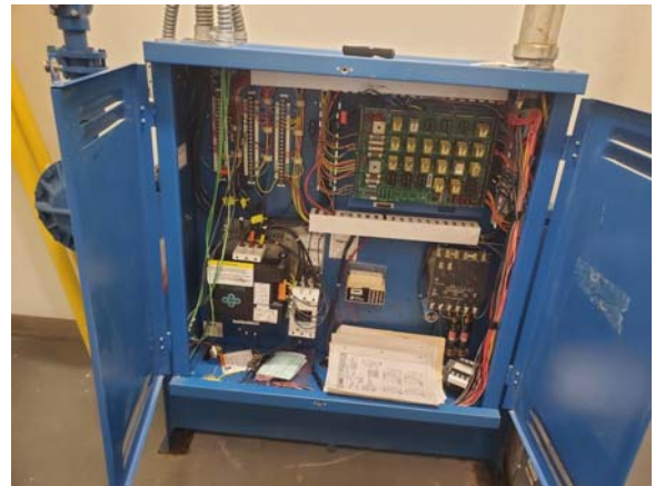
001063e 1/12/2023 Original controls for elevator machine Elevator Machine 1910
