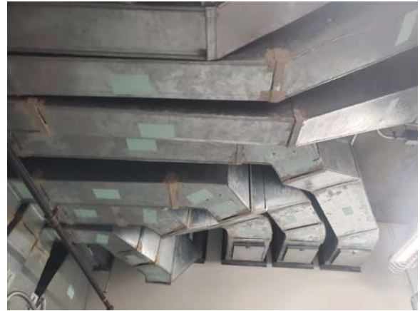
001037e 1/12/2023 Zoned, metal ductwork Mechanical 3904
