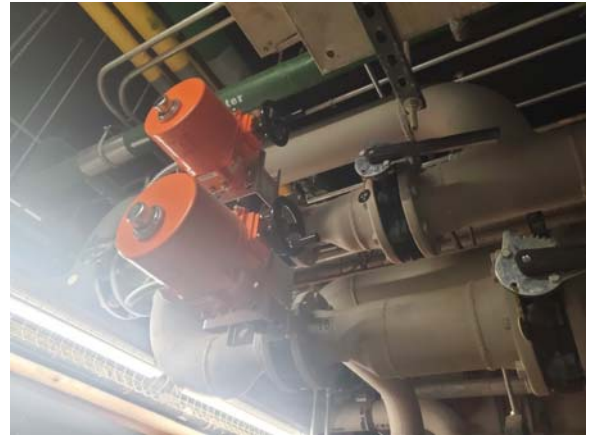
001100e 1/12/2023 Updated controllers for chilled water pipe systems Mechanical B901
