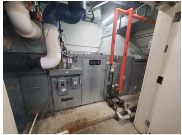
001034e 1/12/2023 Circa 1997 air handler AHU-6 Mechanical 3904
