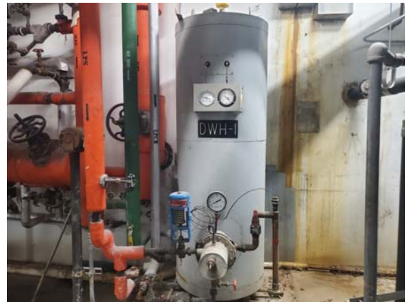
001096e 1/12/2023 Domestic hot water heat exchanger DWH-1 Mechanical B901
