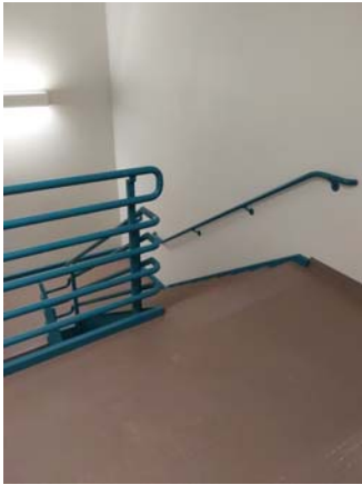
001013a 1/12/2023 Stair tower with noncompliant guardrail Stair 10
