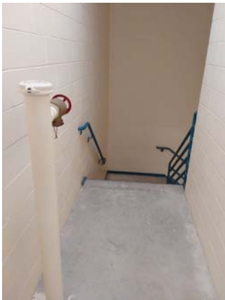
001054a 1/12/2023 Stair with handrail and standpipe Stair 3
