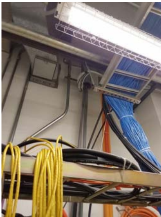
001078a 1/12/2023 Missing fire blocking Room 1911
