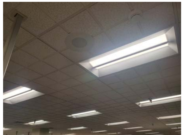
001057e 1/12/2023 Recessed lighting and heat/smoke detector Tech Services 1300
