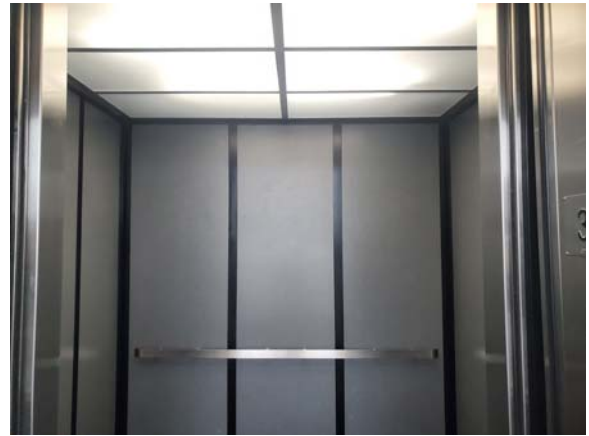
001029e 1/12/2023 Hydraulic elevator 1 Elevator 1
