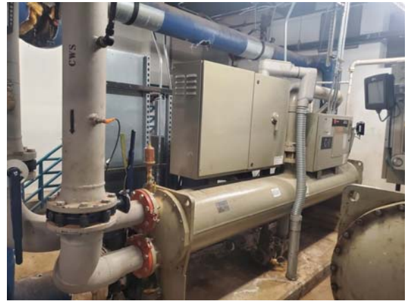
001110e 1/12/2023 Water cooled chiller C-1 Mechanical B901
