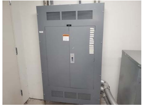
001052e 1/12/2023 208/120 volt, 400 amp panelboard LP22 Mechanical 2911
