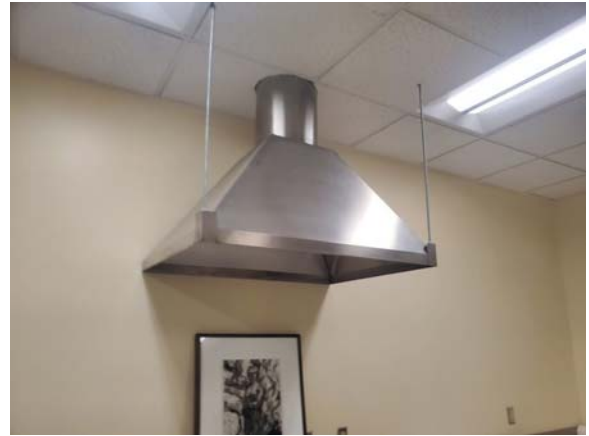
001031e 1/12/2023 Stainless-steel exhaust hood Lab 3405
