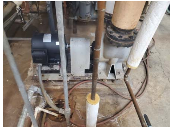
001078e 1/12/2023 Base-mounted hot water pump with new motor Mechanical B909
