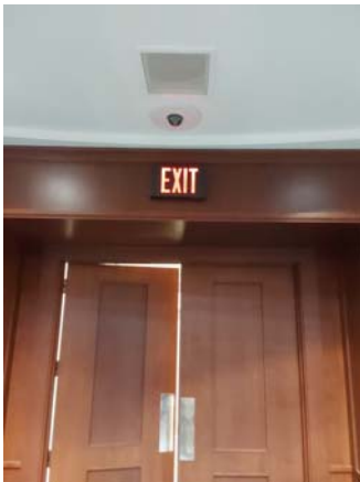
001024a 1/12/2023 Rotunda exit signage at stacks Room 4012
