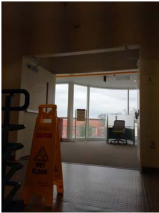
001044a 1/12/2023 Magnetic hold open fire doors Stair 9
