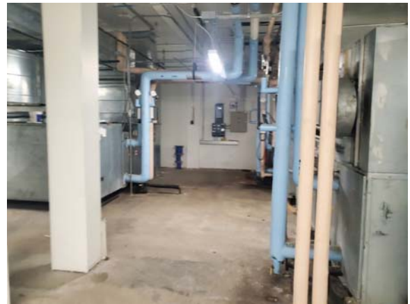
001048e 1/12/2023 Overview of mechanical room and equipment Mechanical 2911
