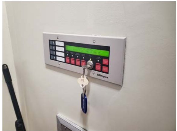
001065e 1/12/2023 Fire alarm system annunciator Lobby 1105
