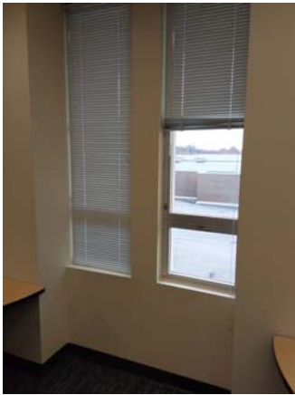
001050a 1/12/2023 Older, single-pane windows Room 3023
