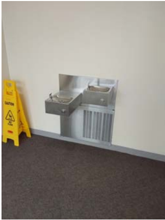
001046a 1/12/2023 Dual-height water fountain Room 3008
