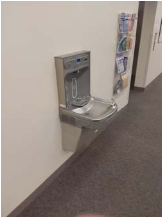
001094a 1/12/2023 Single height water fountain Room 1001
