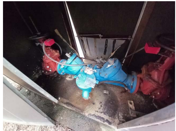
001126e 1/12/2023 Aged fire water backflow device Exterior
