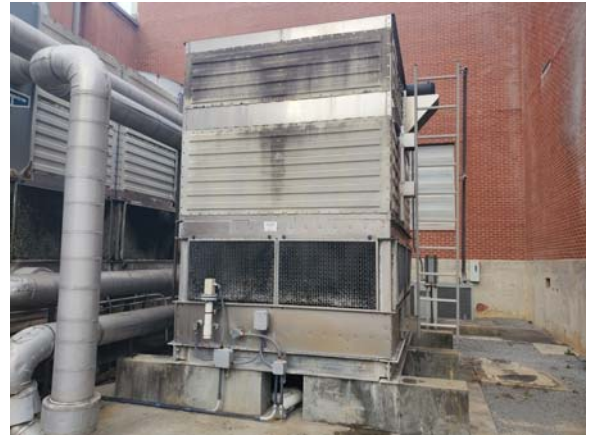
001118e 1/12/2023 Aged cooling tower CT1 Site
