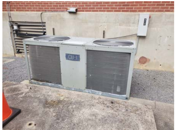
001123e 1/12/2023 Air-cooled condenser CU-1 Site
