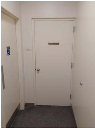
001074a 1/12/2023 Door with noncompliant knob hardware Room 2902
