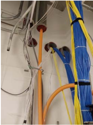
001034a 1/12/2023 Missing fire blocking Room 3906
