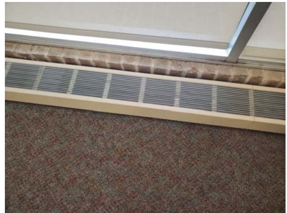
001069e 1/12/2023 Perimeter hydronic heating element Suite 1015
