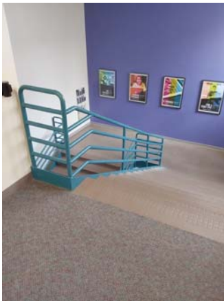
001096a 1/12/2023 Missing handrail extension Stair 3
