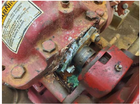
001074e 1/12/2023 Corrosion on fire pump frame and impeller Mechanical B909
