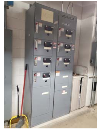
001103e 1/12/2023 Motor control center MCC-1 Mechanical B901
