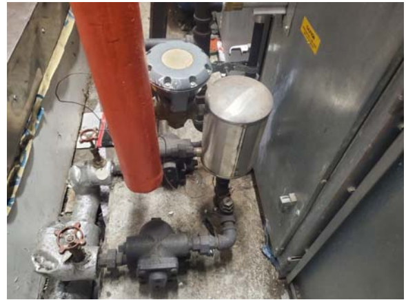
001005e 1/12/2023 Steam injected humidification for AHU-5 Mechanical 4903
