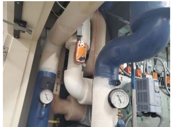
001036e 1/12/2023 Chilled and heating water pipe Mechanical 3904
