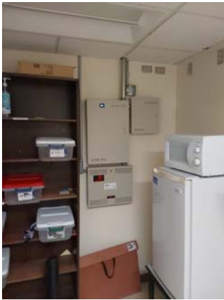
001110a 1/12/2023 Door control panels Room 1902
