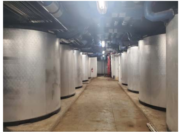
001089e 1/12/2023 Ice storage tanks Mechanical B901
