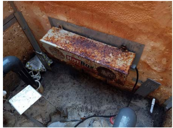
001128e 1/12/2023 Corroded unit heater for backflows Exterior
