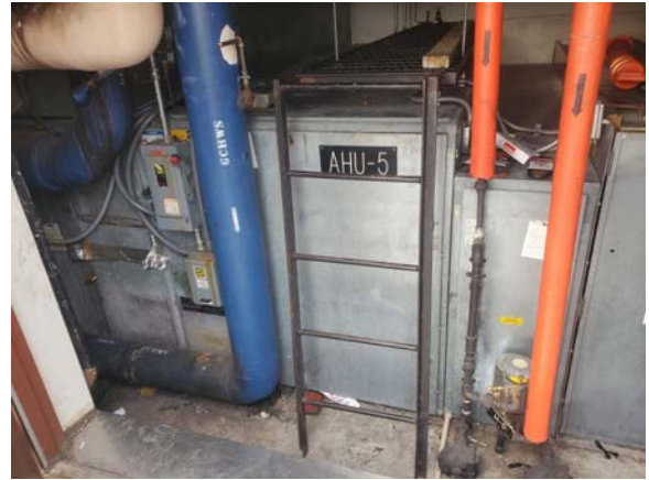
001004e 1/12/2023 Air handler AHU-5 Mechanical 4903
