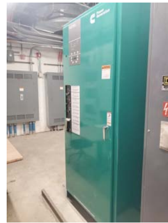
001114e 1/12/2023 600-amp automatic transfer switch Mechanical B901
