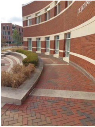
001147a 1/12/2023 Wheelchair ramp without handrail Southeast elevation
