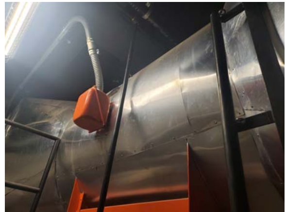
001093e 1/12/2023 Supply air fan for BUAS Mechanical B901
