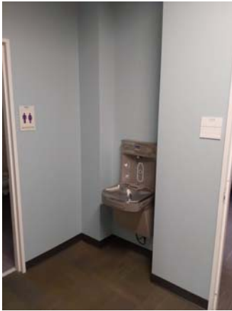
001103a 1/12/2023 Single-height water fountain Room 1047
