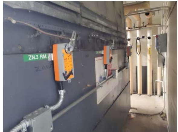
001039e 1/12/2023 Updated controllers for AHU-8 Mechanical 3903
