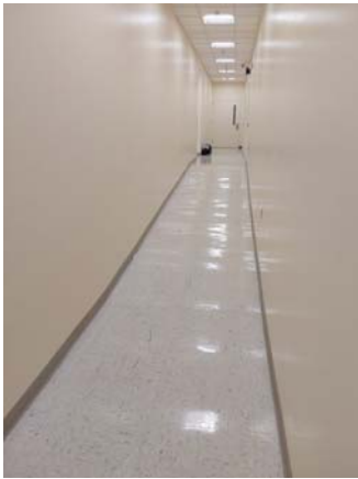
001083a 1/12/2023 Ramp without handrails Room 1092
