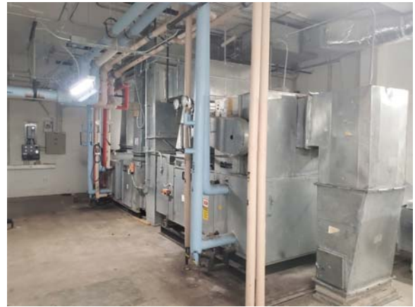
001047e 1/12/2023 Overview of mechanical room and equipment Mechanical 2911
