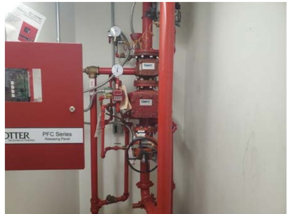
001033e 1/12/2023 Preaction fire suppression system for stacks Mechanical 3407
