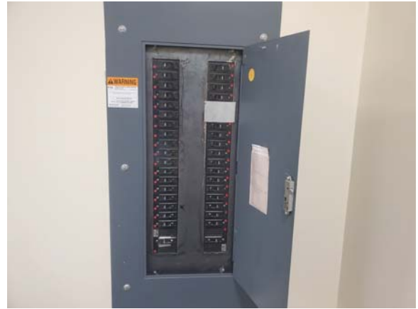
001055e 1/12/2023 Aged secondary electric panelboard Teaching resources 2020
