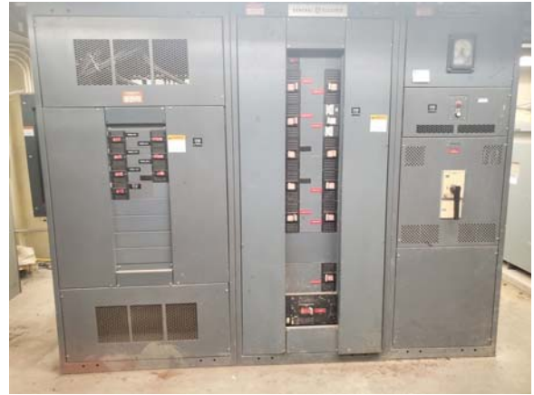
001076e 1/12/2023 Aged 2,000-amp switchboard SSB Mechanical B909
