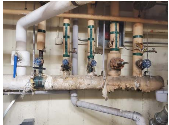
001084e 1/12/2023 Original cold water header station with damaged insulation Mechanical B909
