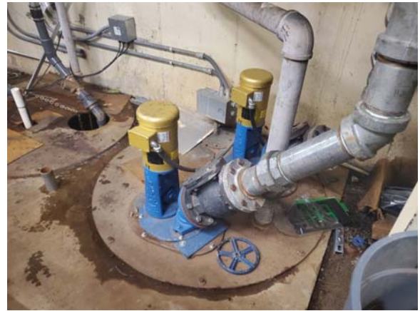
001083e 1/12/2023 Duplex sump pump system Mechanical B909
