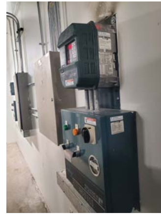
001050e 1/12/2023 Variable speed drive for AHU-3 Mechanical 2911
