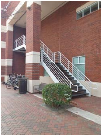
001130a 1/12/2023 South stair with missing handrail East elevation
