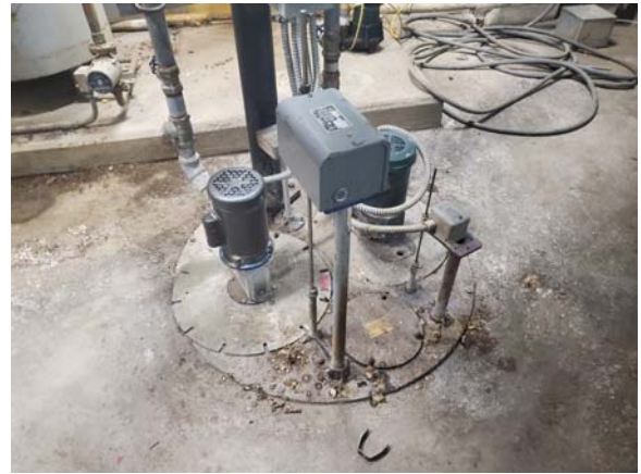
001095e 1/12/2023 Duplex sewage ejection station Mechanical B901
