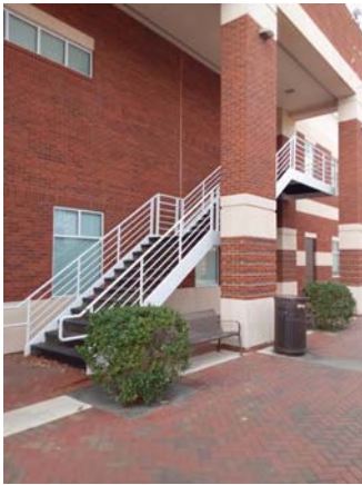
001131a 1/12/2023 North stair with missing handrail East elevation
