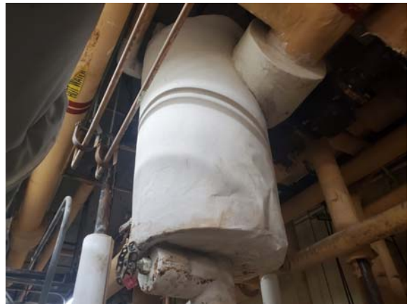
001081e 1/12/2023 Hot water system air separator Mechanical B909
