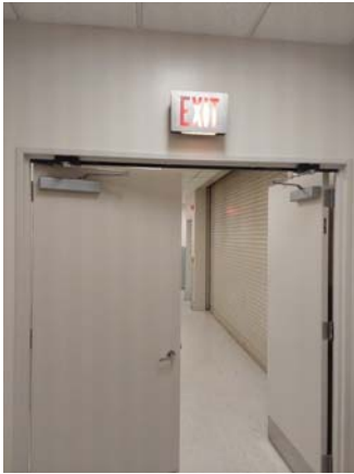
001079a 1/12/2023 Fire doors with noncompliant hardware Room 1080
