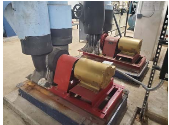
001105e 1/12/2023 Chilled water system pumps Mechanical B901
