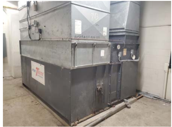
001038e 1/12/2023 Circa 1976 air handler AHU-8 that has been modernized Mechanical 3903
