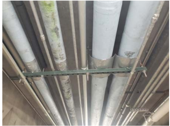
001115e 1/12/2023 Various utility piping Mechanical service tunnel
