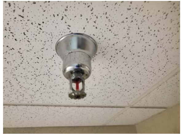
001017e 1/12/2023 Fire sprinkler head Recept. 4003
