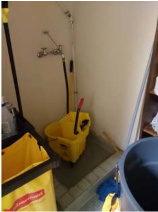
001115a 1/12/2023 Mop sink Room B909
