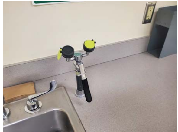
001032e 1/12/2023 Emergency eyewash/drench hose plumbing fixture Lab 3405
