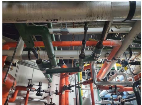
001099e 1/12/2023 Various distribution system piping Mechanical B901
