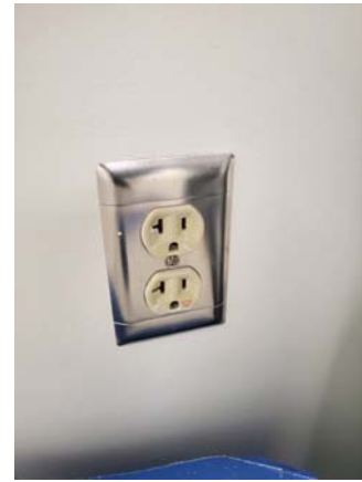
001010e 1/12/2023 Standard secondary electrical system outlet Data 4901
