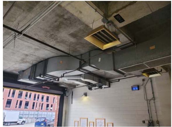
001059e 1/12/2023 Infrared unit heaters and inline exhaust fans Loading Dock 1211
