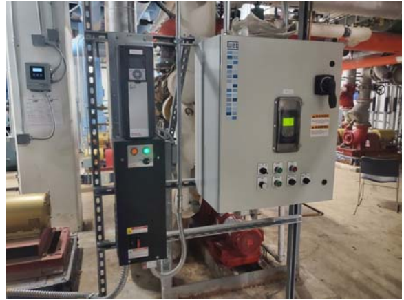
001106e 1/12/2023 Chilled water pump variable speed drives Mechanical B901
