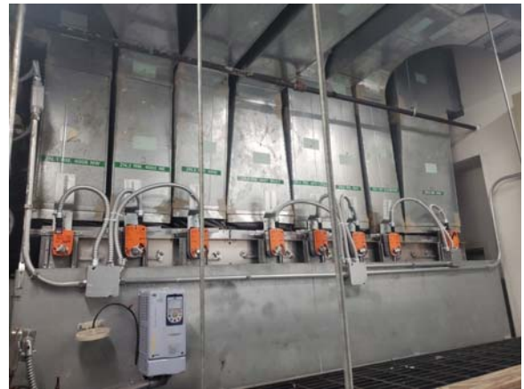
001006e 1/12/2023 Modernized electronic zone controller and VSD for AHU-5 Mechanical 4903
