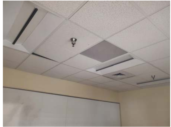
001046e 1/12/2023 2x4 lighting and fire sprinkler head Group Study 2213
