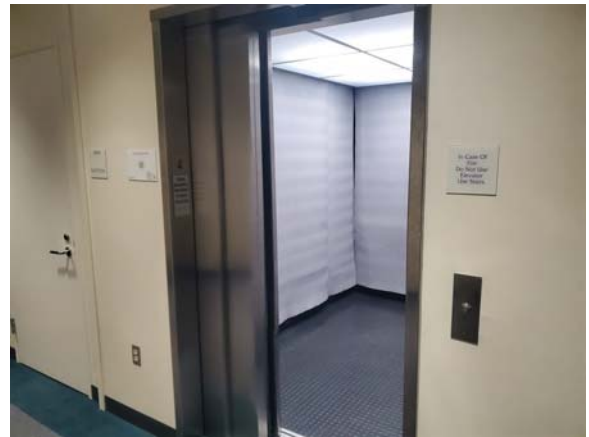
001021e 1/12/2023 Hydraulic elevator 2 Elevator 2
