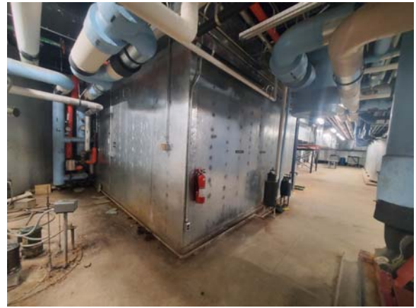
001092e 1/12/2023 Main building air handler BUAS Mechanical B901
