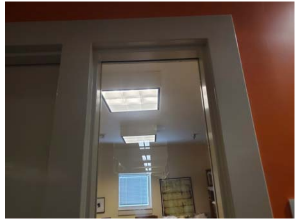
001026e 1/12/2023 Circa 1997 2x2 surface mounted lighting in offices Office 3308
