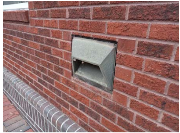
001130e 1/12/2023 Recessed exterior light fixture Exterior
