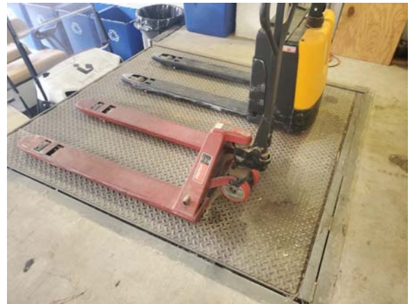
001060e 1/12/2023 Hydraulic dock levelers Loading Dock 1211
