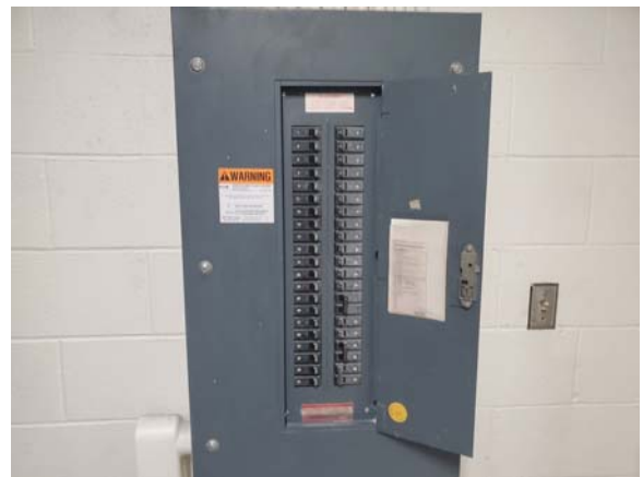
001042e 1/12/2023 Circa 1976 secondary electric system panelboard Mechanical 3903
