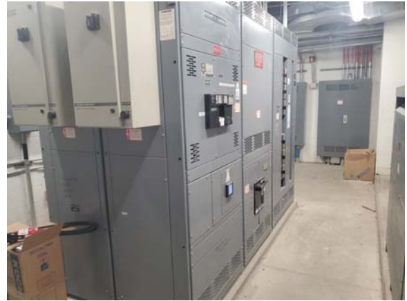
001112e 1/12/2023 2,500-amp main switchboard MSB2 Mechanical B901
