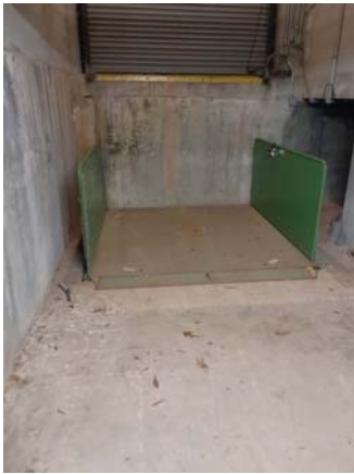
001125a 1/12/2023 Freight lift Room B900
