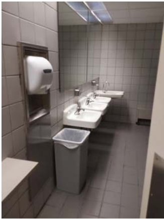
001053a 1/12/2023 Wall-hung lavatories and ceramic wall and floor tile Room 3001
