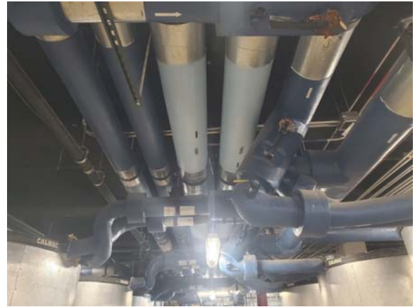
001088e 1/12/2023 Glycol chilled water system piping Mechanical B901
