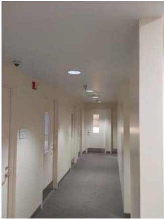
001076a 1/12/2023 Corridor without exit signage Room 2118
