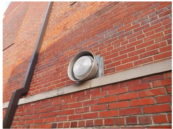
033066e Steam kettle hood exhaust fan Exterior 1/10/2023
