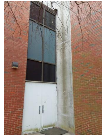
033080a 1/10/2023 Deteriorated steel mullions with grime on wall West elevation
