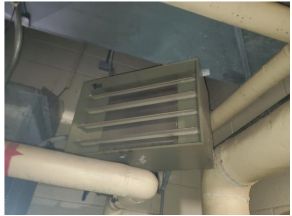
033052e 1/10/2023 Aged hydronic unit heater Mechanical 126
