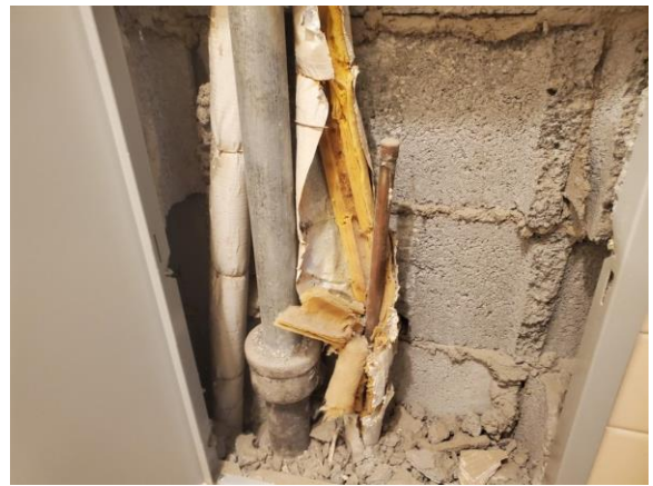
033018e 1/10/2023 Aged supply and waste piping Room 203
