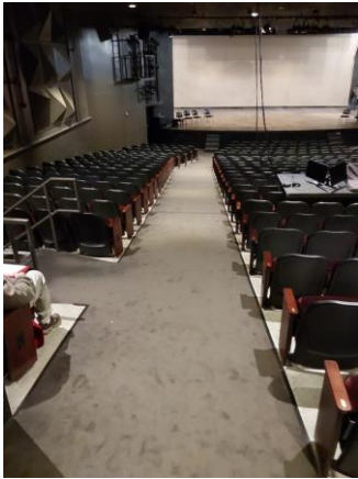
033014a 1/10/2023 Missing aisle handrail Room 209
