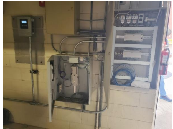
033063e 1/10/2023 Updated HVAC control system components Mechanical 126
