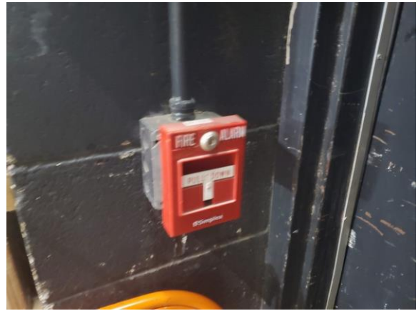
033002e 1/10/2023 Fire alarm pull station Stage 209
