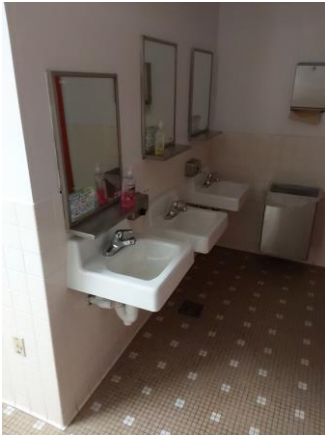
033067a 1/10/2023 Wall-hung lavatories with mirrors Room 108
