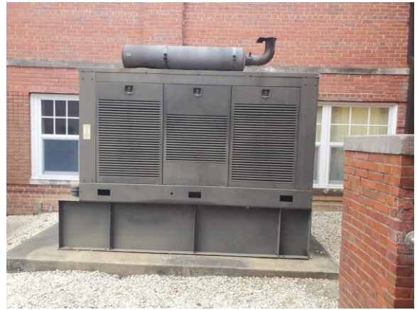
033070e 1/10/2023 Diesel-fired emergency generator Exterior
