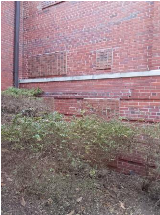
033089a 1/10/2023 Damaged brick on wall East elevation
