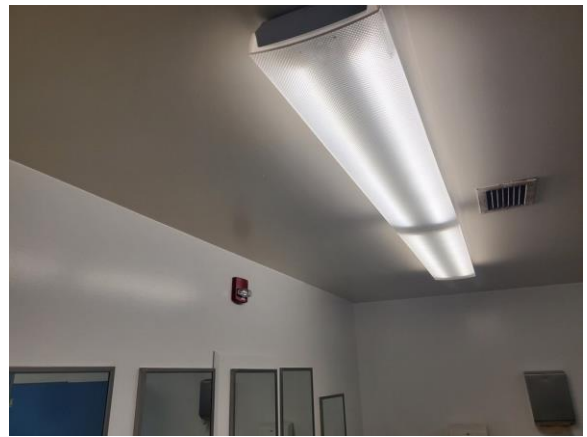
033036e 1/10/2023 Surface-mounted lighting Restroom 105
