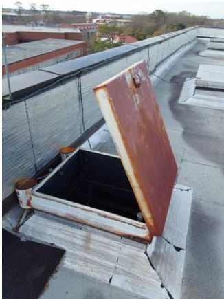
033003a 1/10/2023 Rusted roof hatch Stage roof
