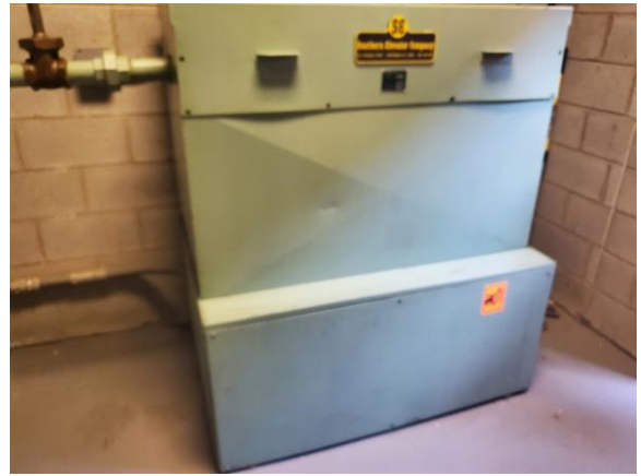
033022e 1/10/2023 Aged hydraulic elevator machine Elevator machine room 128
