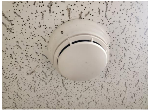
033037e 1/10/2023 Smoke/heat detector Restroom 105
