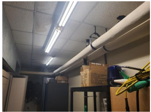
033006e 1/10/2023 Aged lighting and distribution piping Dimmer room 214
