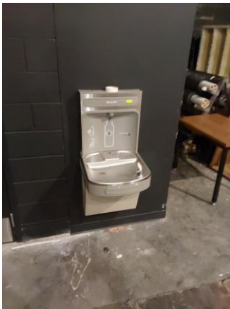
033006a 1/10/2023 Single water fountain Room 209
