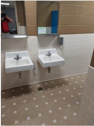
033055a 1/10/2023 Wall-hung lavatories Room 129
