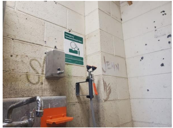
033016e 1/10/2023 Emergency eyewash/drench hose Room 204
