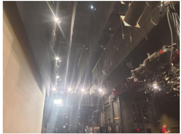
033004e 1/10/2023 Overview of theater lighting Stage 209
