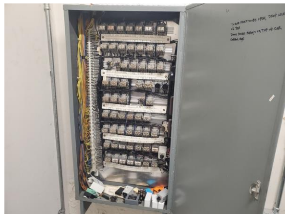
033039e 1/10/2023 Aged elevator machine controls Elevator machine room 103
