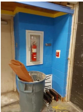
033039a 1/10/2023 Fire extinguisher cabinet and alarm Room 101
