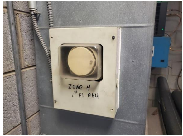
033026e 1/10/2023 Aged duct detector Mechanical 127
