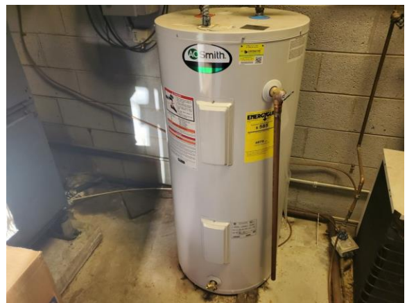
033033e 1/10/2023 Electric domestic water heater Mechanical 127
