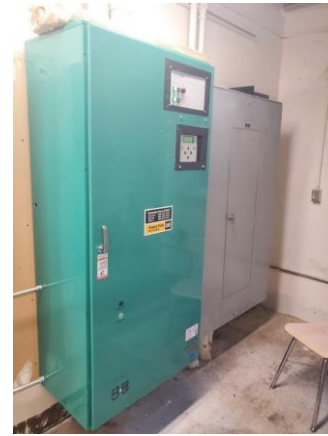
033047e 1/10/2023 208V, 800A automatic transfer switch Mechanical 111
