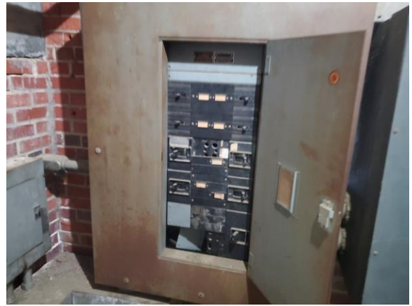
033043e 1/10/2023 Original electrical switchboard Room 112A
