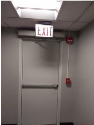
033070a 1/10/2023 Exit door with panic hardware signage Room 101
