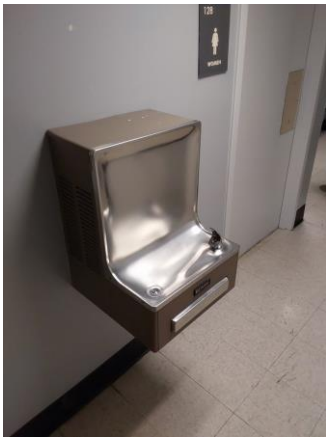
033054a 1/10/2023 Noncompliant water fountain Room 122
