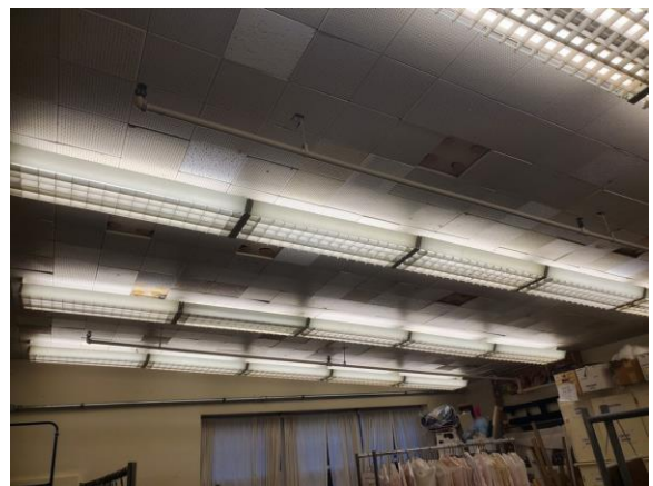
033042e 1/10/2023 Aged, open cell lighting Room 112
