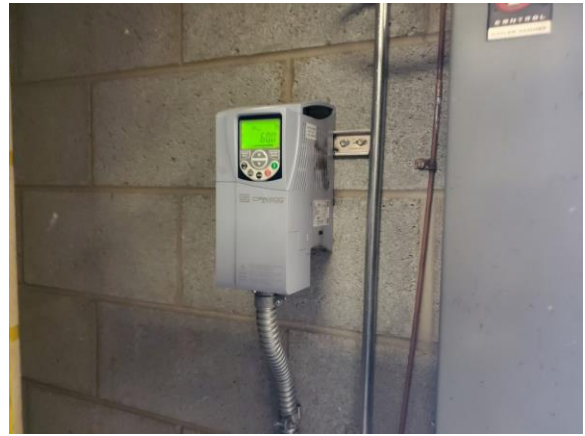
033029e 1/10/2023 Variable speed drive for air handler Mechanical 127
