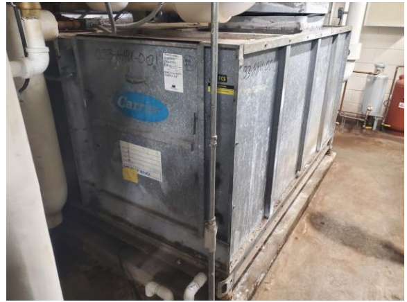
033056e 1/10/2023 Air handler Mechanical 126
