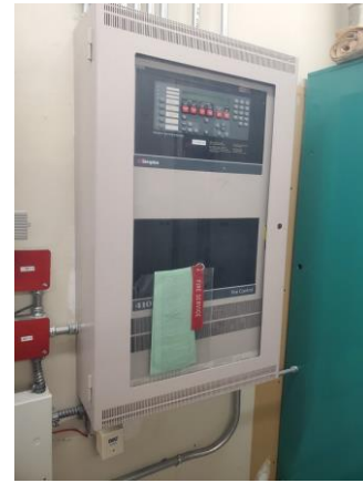
033046e 1/10/2023 Main fire alarm control panel Mechanical 111
