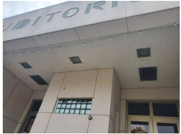
033068e 1/10/2023 Aged and corroded recessed exterior lights Exterior
