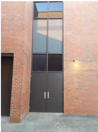
033045a 1/10/2023 Exterior hollow-metal door Room 121
