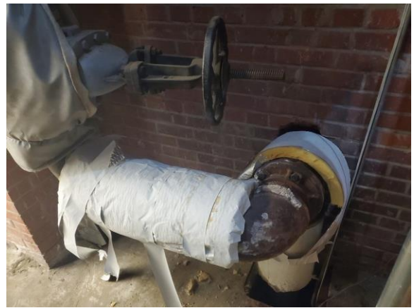
033045e 1/10/2023 Leaking main steam pipe Room 112A
