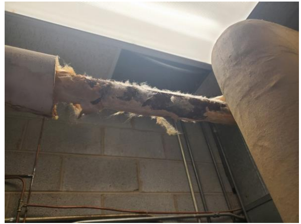
033025e 1/10/2023 Corroded pipe and damaged insulation Mechanical 127
