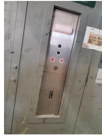
033014e 1/10/2023 Freight elevator control Freight elevator
