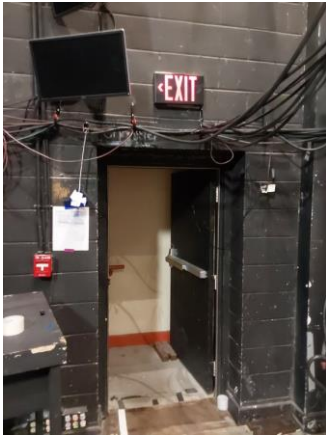
033010a 1/10/2023 Exit door with typical panic hardware and signage Room 209
