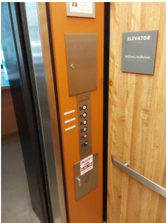
033021a 1/10/2023 Noncompliant elevator control board Room 202
