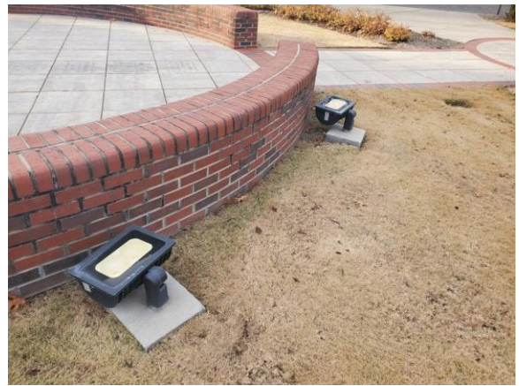
033069e 1/10/2023 Upward illuminating site lighting Exterior
