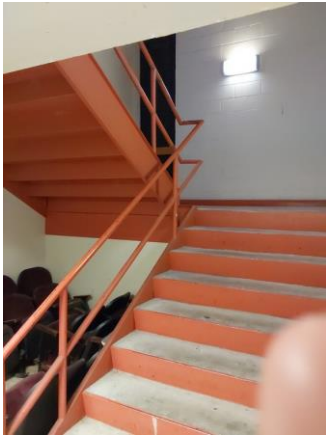
033075a 1/10/2023 Noncompliant stair handrail Room 121
