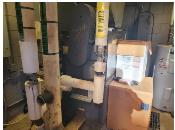
033024e 1/10/2023 Trane air handler Mechanical 127
