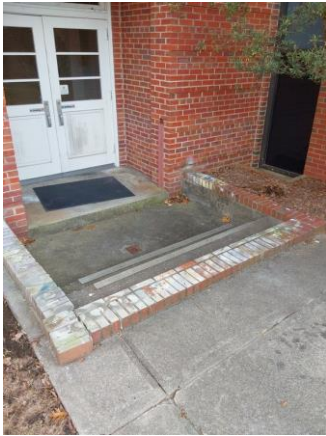
033071a 1/10/2023 Trip hazard and drainage issue Room 110
