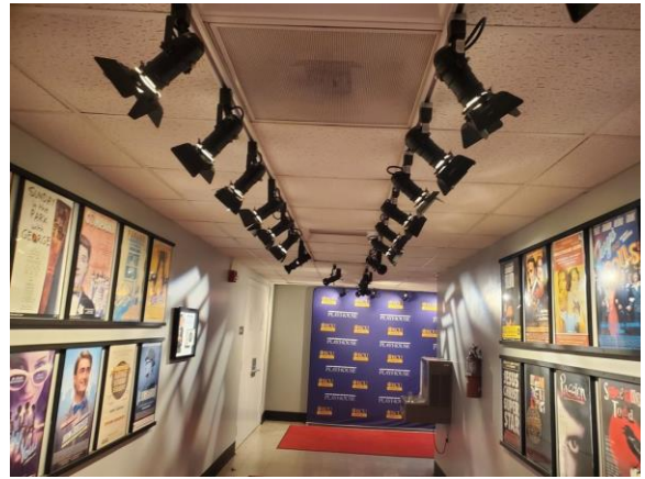
033035e 1/10/2023 Overview of systems Corridor 106
