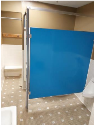
033058a 1/10/2023 Toilet partition Room 129
