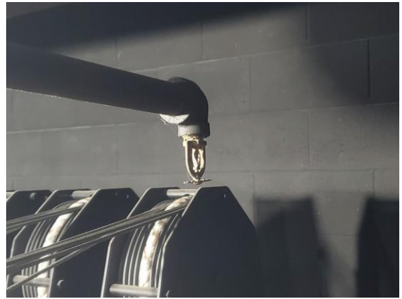
033001e 1/10/2023 Fire suppression system sprinkler head Auditorium mezzanine
