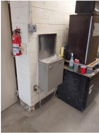
033026a 1/10/2023 Noncompliant water fountain 2-E-1
