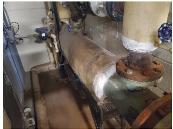
033051e 1/10/2023 Shell-and-tube heat exchanger Mechanical 126
