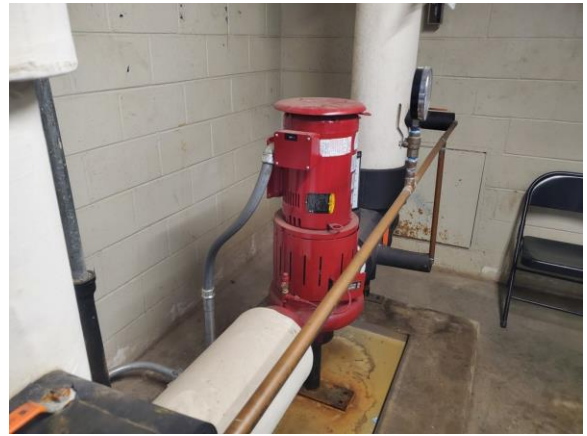
033062e 1/10/2023 Chilled water pump Mechanical 126
