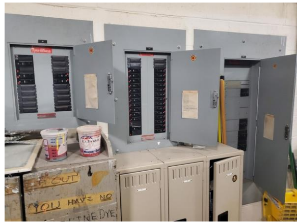
033021e 1/10/2023 1980s vintage secondary electrical equipment Scene shop room 101
