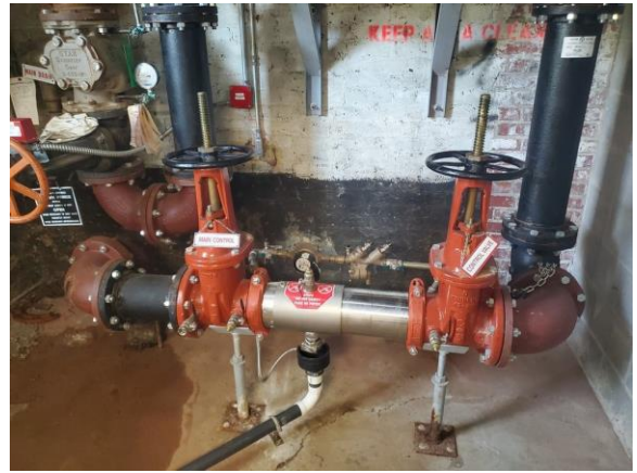
033040e 1/10/2023 Fire system backflow with bypass Sprinkler riser room 135
