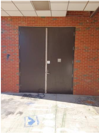
033035a 1/10/2023 Hollow-metal door Room 131
