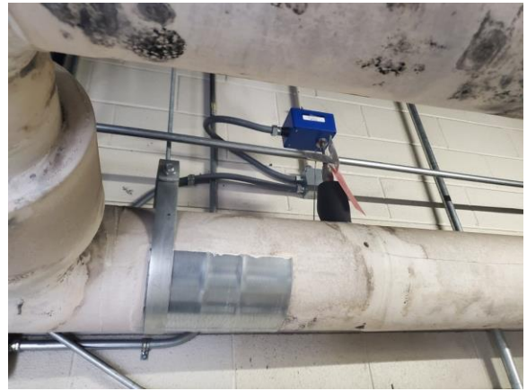
033061e 1/10/2023 Updated controls on distribution piping Mechanical 126
