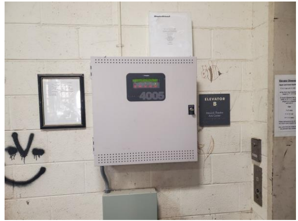
033020e 1/10/2023 Fire alarm control panel for Scene shop Scene shop 2-E-2
