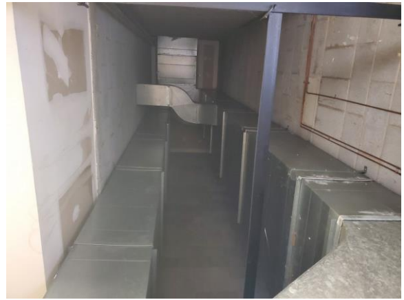
033034e 1/10/2023 Metal HVAC distribution ductwork Mechanical 127
