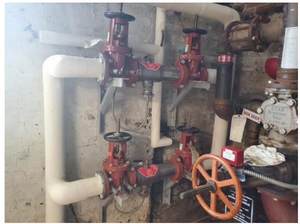
033041e 1/10/2023 Domestic water system backflow devices Sprinkler riser room 135
