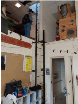
033031a 1/10/2023 Partial roof ladder safety hazard 2-E-1
