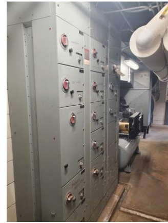
033058e 1/10/2023 Aged motor control center Mechanical 126
