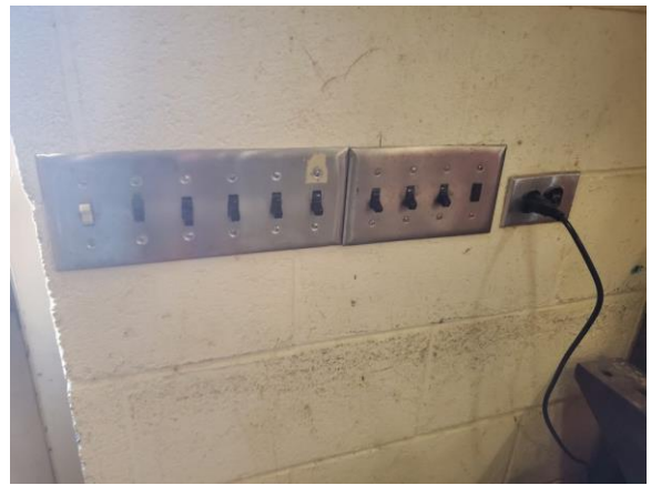
033015e 1/10/2023 Aged light switches Scene shop 2-E-2
