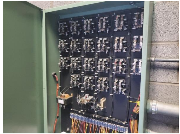
033023e 1/10/2023 Aged elevator machine controls Elevator machine room 128
