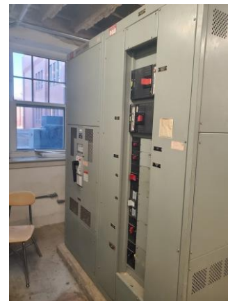
033048e 1/10/2023 2000A switchboard with main breaker Mechanical 111
