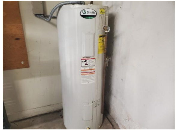
033049e 1/10/2023 Electric domestic water heater Mechanical 111
