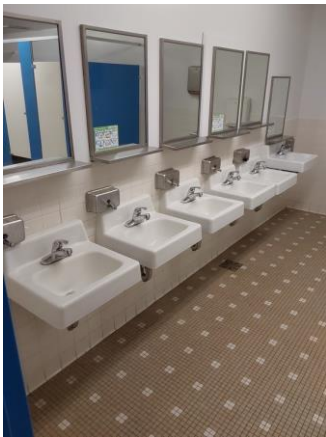
033063a 1/10/2023 Wall-hung lavatories Room 105
