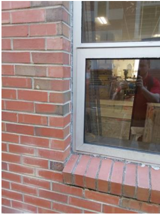
033043a 1/10/2023 Deteriorated seals on shop windows Room 101
