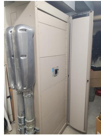
033007e 1/10/2023 800-amp dimmer panel Dimmer room 214
