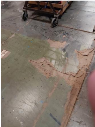
033004a 1/10/2023 Deteriorating stage floor Room 209
