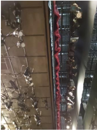
033005a 1/10/2023 Stage fire curtain Room 209
