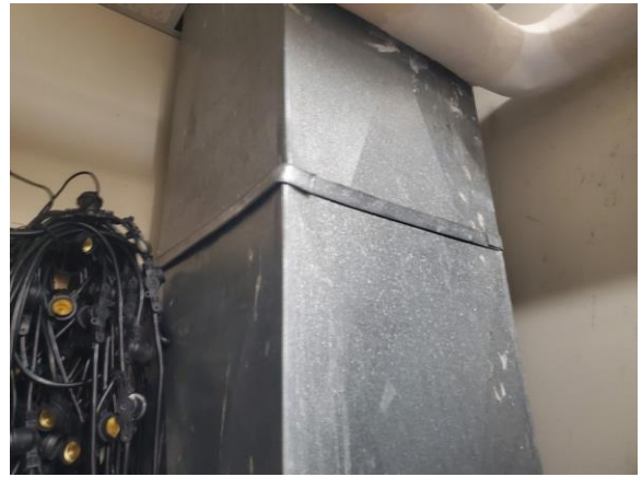
033008e 1/10/2023 Metal HVAC ductwork Dimmer room 214
