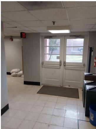
033060a 1/10/2023 Exterior door with old panic hardware and exit signage Room 110
