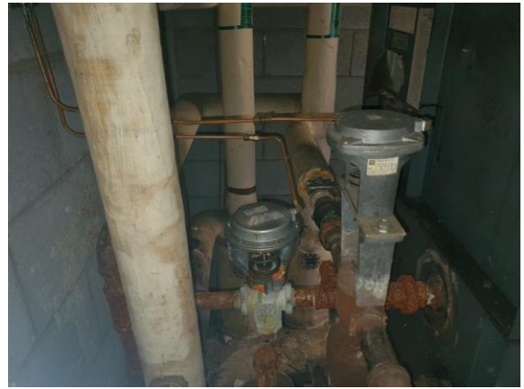
033031e 1/10/2023 Aged pneumatic controls and corroded pipe Mechanical 127
