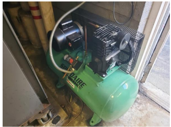
033027e 1/10/2023 Reciprocating air compressor Mechanical 127
