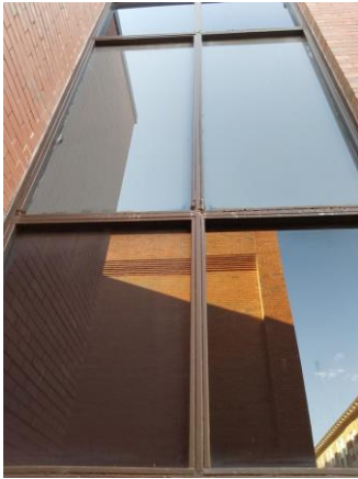
033046a 1/10/2023 Deteriorated steel mullions Room 121
