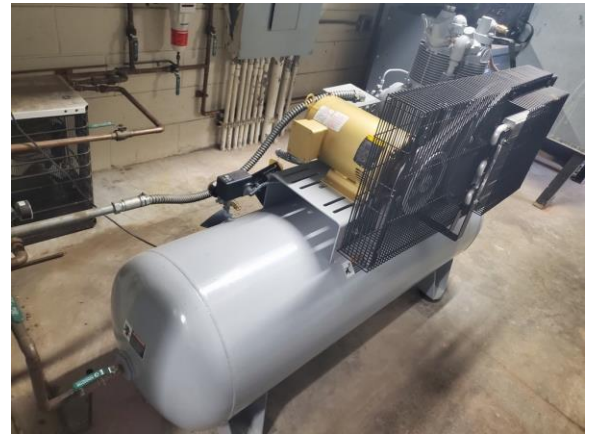
033059e 1/10/2023 Reciprocating air compressor Mechanical 126
