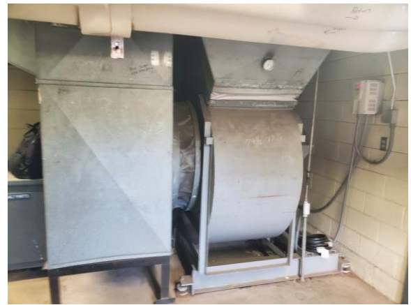
033060e 1/10/2023 Utility set return fan #5 Mechanical 126
