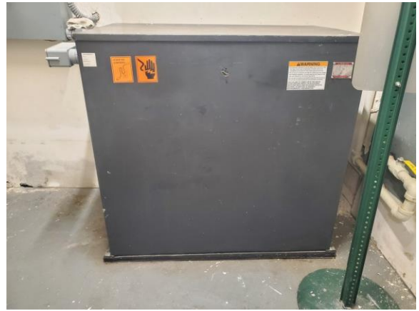
033038e 1/10/2023 Hydraulic elevator machine Elevator machine room 103
