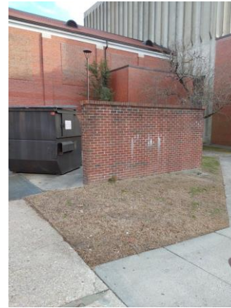
033082a 1/10/2023 Efflorescence on dumpster walls West elevation
