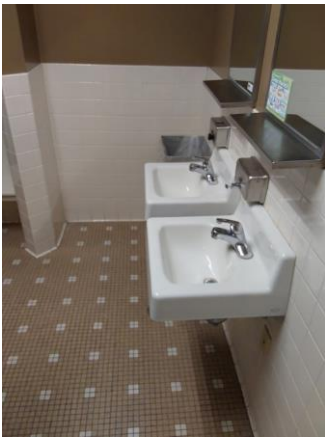
033051a 1/10/2023 Wall-hung lavatories Room 128
