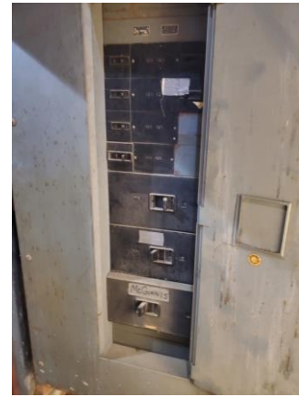
033044e 1/10/2023 Original electrical switchboard Room 112A
