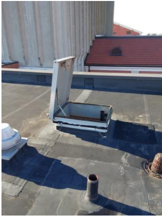
033028a 1/10/2023 Roof hatch with missing fall protection 2-E-1
