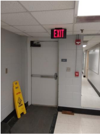
033050a 1/10/2023 Exit door with panic hardware and signage Room 122
