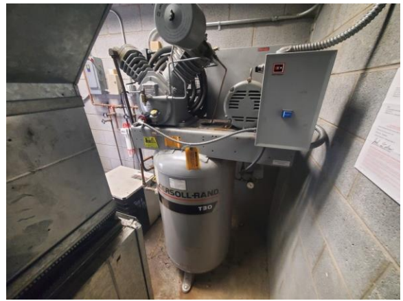
033032e 1/10/2023 Reciprocating air compressor Mechanical 127
