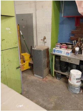
033038a 1/10/2023 Noncompliant water fountain Room 101
