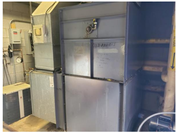
033030e 1/10/2023 Trane air handler Mechanical 127
