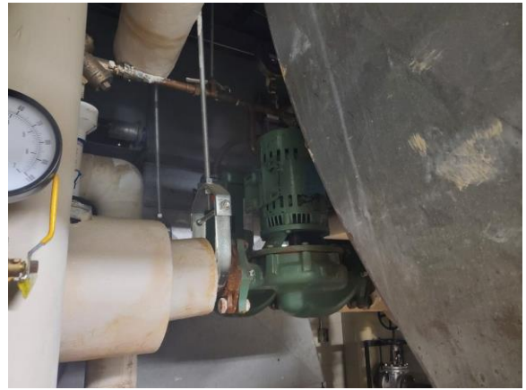
033055e 1/10/2023 Heating water pump Mechanical 126
