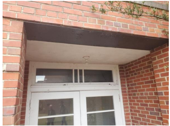
033065e Aged surface mounted light fixture Exterior 1/10/2023
