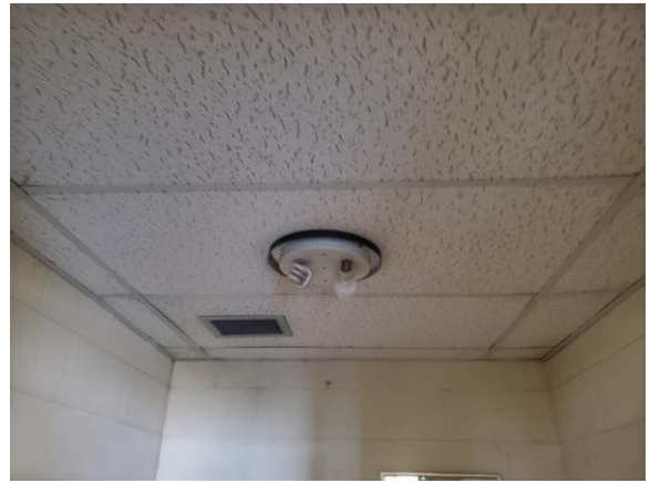
033017e 1/10/2023 Aged surface-mounted light fixture Room 203
