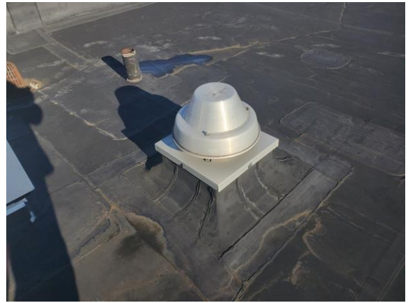
033019e 1/10/2023 Typical rooftop exhaust fan Scene shop roof
