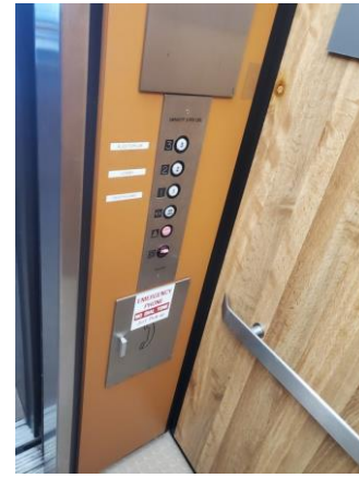
033011e 1/10/2023 Passenger elevator controls Elevator
