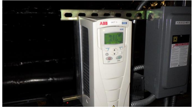
047019e 1/26/2023 FCU#5 supply fan VFD Attic (above 2300)
