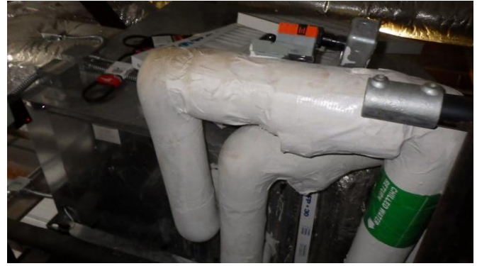
047022e 1/26/2023 HVAC distribution network chilled water piping Attic (above 2300)
