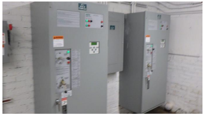
047092e 1/26/2023 Emergency power ATS-1 and ATS-2 Electrical room G401
