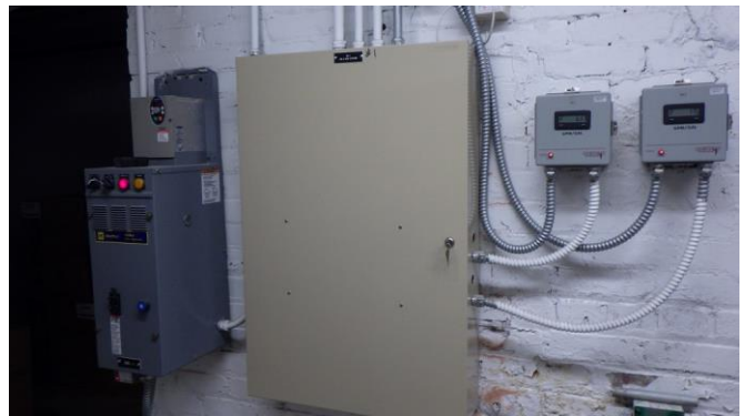
047035e 1/26/2023 HVAC controls panel, flow (energy) meters Mechanical room G520
