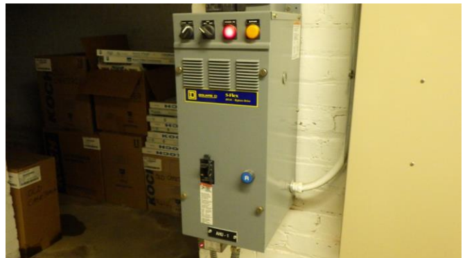
047038e 1/26/2023 AH#1 supply fan VFD Square D Mechanical room G520
