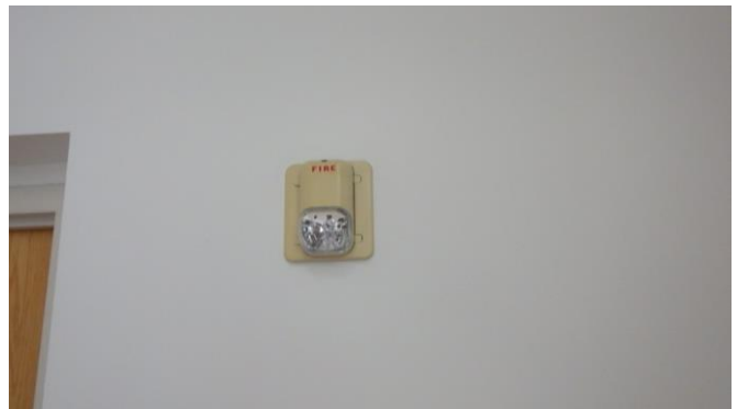
047008e 1/26/2023 Fire alarm system horn strobe Second floor, stair A
