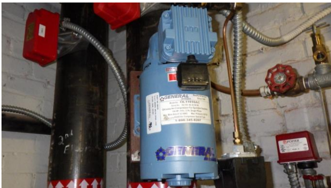
047045e 1/26/2023 Fire suppression system main risers Mechanical room G520
