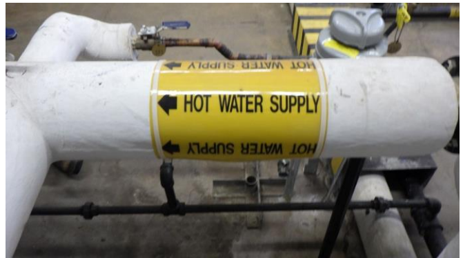
047032e 1/26/2023 HVAC distribution network heating hot water piping Mechanical room G520
