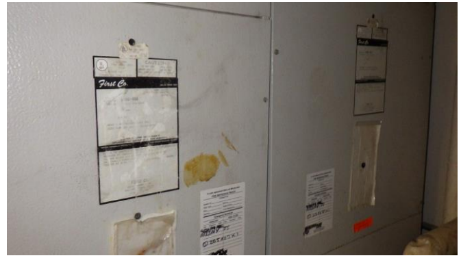
047066e 1/26/2023 Old built-in place air handler Mechanical room G137
