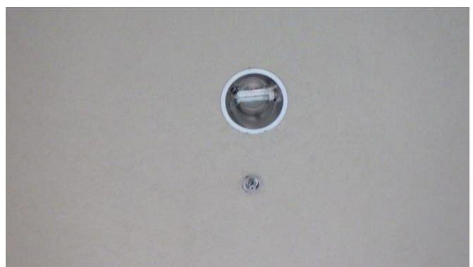
047082e 1/26/2023 Recessed CFL exterior light fixture North side covered walk
