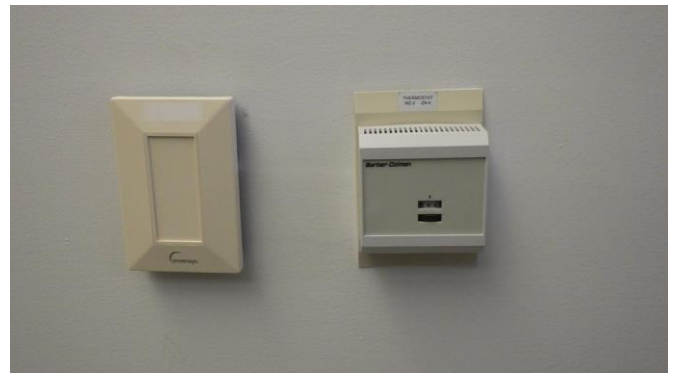
047023e 1/26/2023 HVAC sensor and thermostat Corridor 2200D
