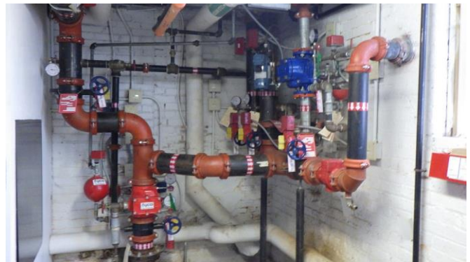
047044e 1/26/2023 AH#2 supply fan VFD Square D Mechanical room G520
