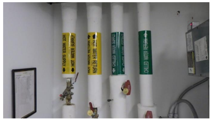
047050e 1/26/2023 Fan coil unit FC#1 Mechanical room G403C
