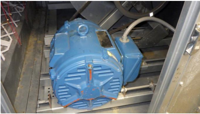
047061e 1/26/2023 AH#4 supply fan motor Mechanical room G301
