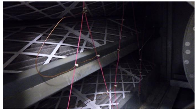
047062e 1/26/2023 AH#4 filtration section Mechanical room G301
