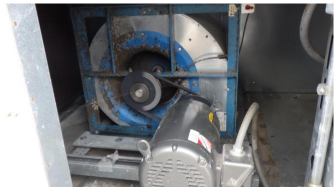
047003e 1/26/2023 Blower box for RT#1 Roof, south side
