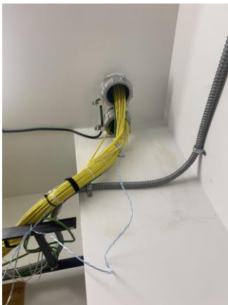
047015a 1/26/2023 Penetration through ceiling Data closet
