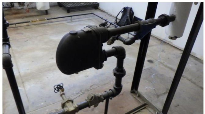
047030e 1/26/2023 HVAC distribution network steam trap Mechanical room G520
