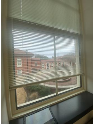
047016a 1/26/2023 Dual-pane, metal frame window Tutor room
