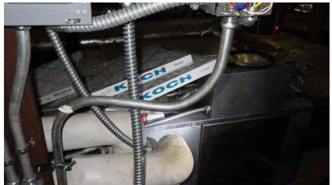
047020e 1/26/2023 FCU #6 Attic (above 2300)
