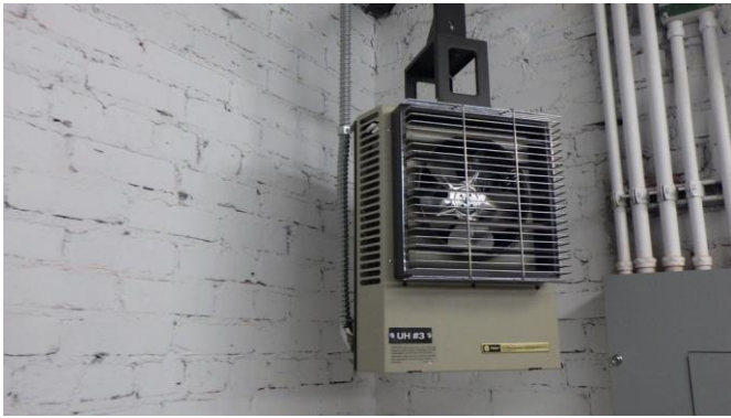
047091e 1/26/2023 Electric unit heater UH#3 Electrical room G401
