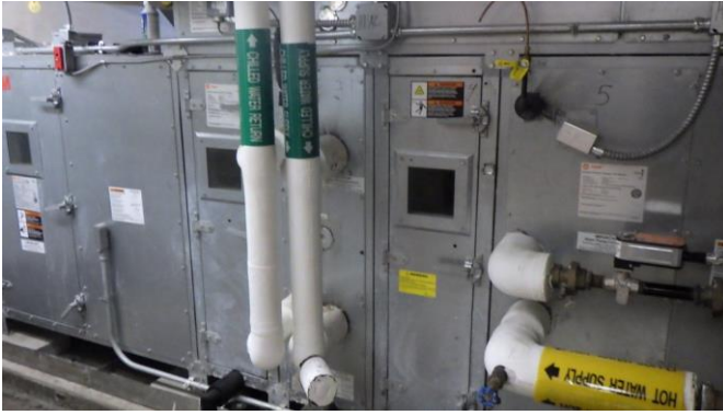
047059e 1/26/2023 Indoor AH#4 Mechanical room G301
