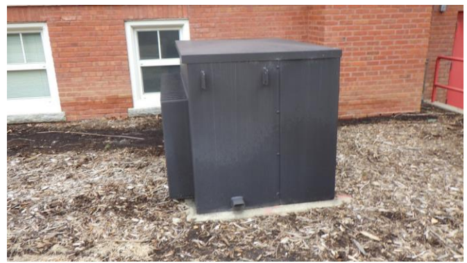
047086e 1/26/2023 Primary electrical distribution transformer West exterior
