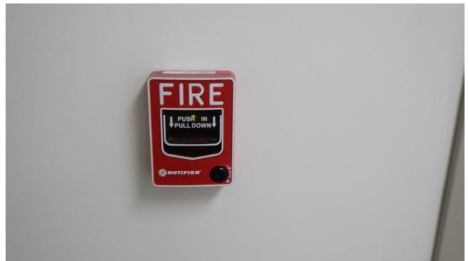
047014e 1/26/2023 Fire alarm system manual pull station Second floor, stair B
