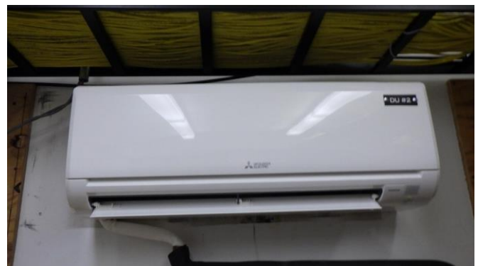
047018e 1/26/2023 Ductless split system evaporative unit DU#2 Communications 2210
