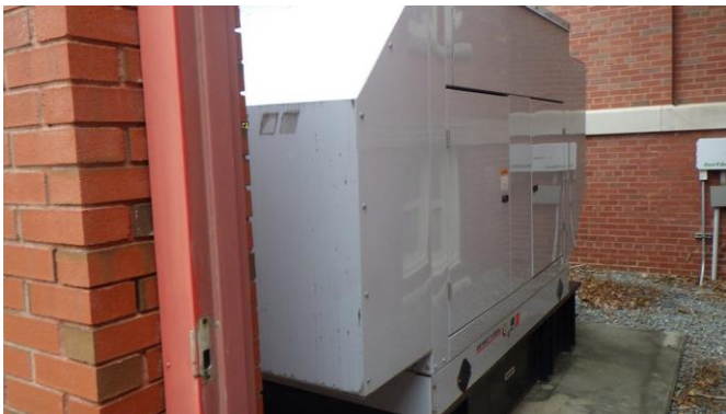
047093e 1/26/2023 Diesel fuel emergency generator West exterior
