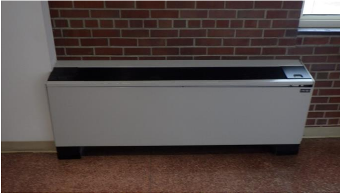
047077e 1/26/2023 Fan coil unit #2 Second floor, stair A
