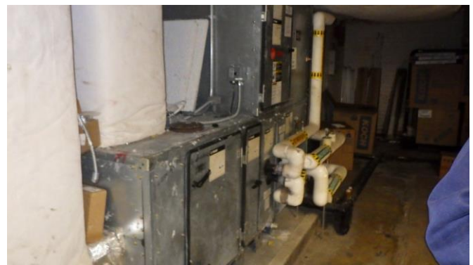
047068e 1/26/2023 Indoor AH#11 Mechanical room G134
