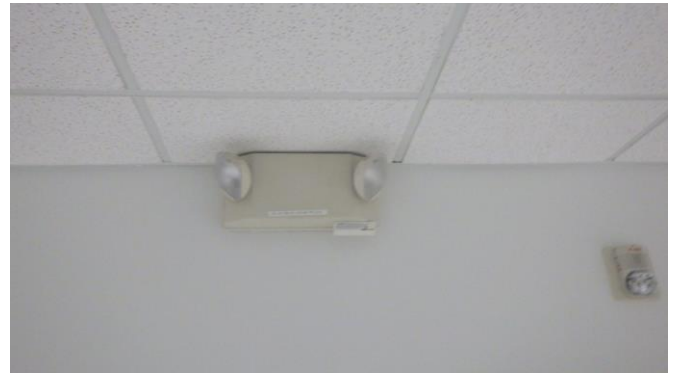
047072e 1/26/2023 Battery backup emergency exit light fixture Corridor G100A
