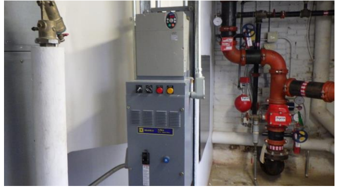
047043e 1/26/2023 AH#2 supply fan VFD, Square D Mechanical room G520
