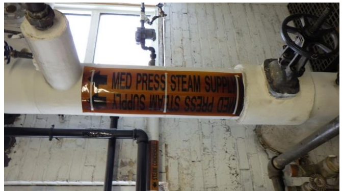
047026e 1/26/2023 Campus steam distribution network Mechanical room G520
