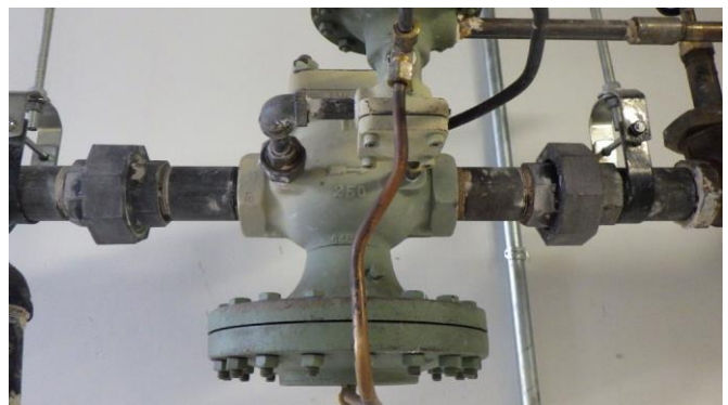
047027e 1/26/2023 Medium to service pressure PRV Mechanical room G520
