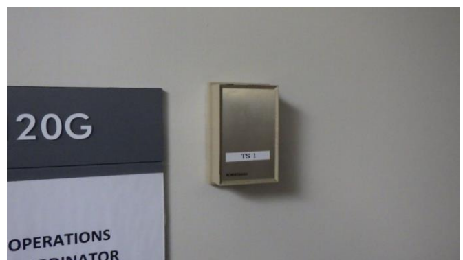
047076e 1/26/2023 HVAC sensor Office suite G120
