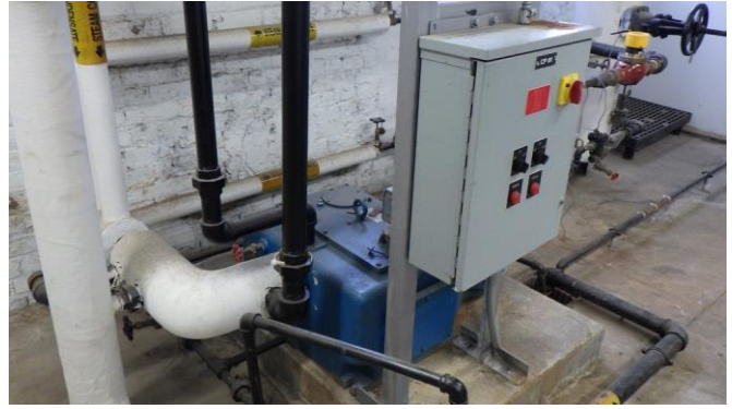
047034e 1/26/2023 Steam electric duplex condensate receiver CP#1 Mechanical room G520
