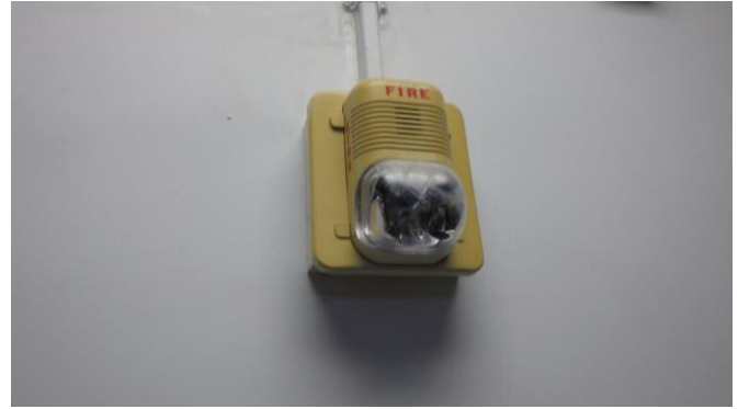
047004e 1/26/2023 Fire alarm system horn strobe Men's restroom 2101
