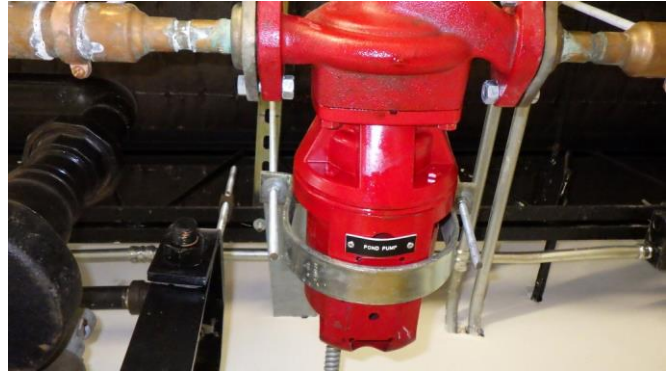
047028e 1/26/2023 Fountain pump Mechanical room G520
