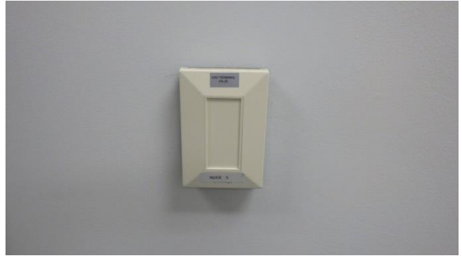
047013e 1/26/2023 HVAC sensor Office suite 2100
