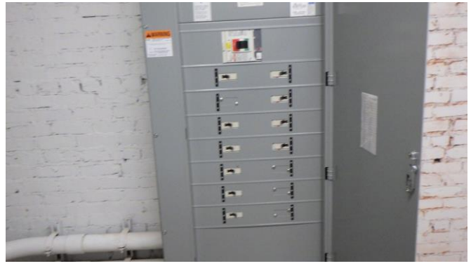
047090e 1/26/2023 Main electrical distribution panel DP Electrical room G401
