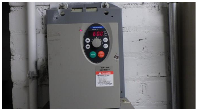
047039e 1/26/2023 AH#1 supply fan VFD Square D Mechanical room G520
