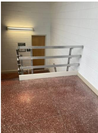
047003a 1/26/2023 CMU walls, terrazzo floor, noncompliant guardrail Stairwell
