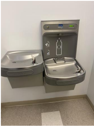
047022a 1/26/2023 Dual-level drinking fountain Corridor
