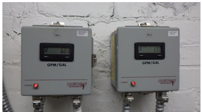
047036e 1/26/2023 HVAC chilled and heating hot water flow (energy) meters Mechanical room G520
