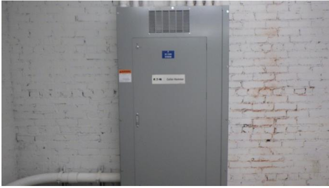
047089e 1/26/2023 Main electrical distribution panel DP Electrical room G401
