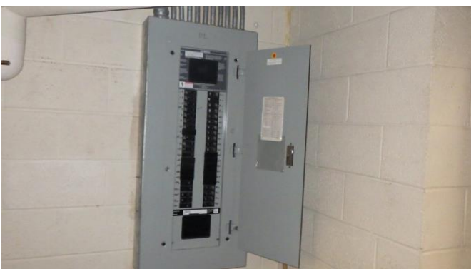
047069e 1/26/2023 Secondary electrical distribution panel DL Mechanical room G134
