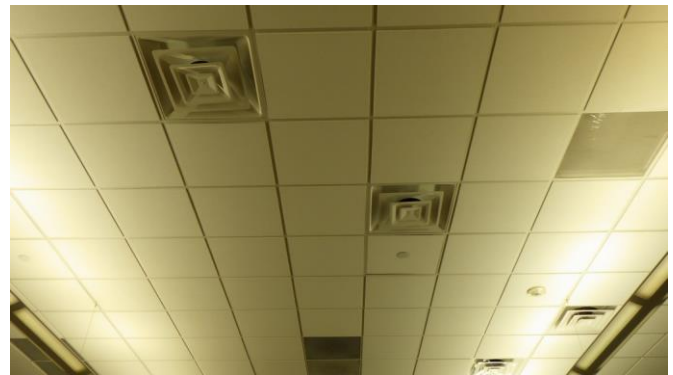
047017e 1/26/2023 Central HVAC air distribution supply grille, concealed fire suppression sprinkler head Tutoring 2300
