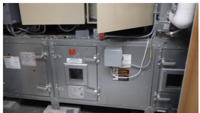
047052e 1/26/2023 Indoor AH#3 Mechanical room G410
