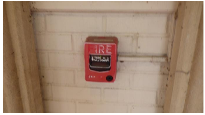
047084e 1/26/2023 Fire alarm system manual pull station North side covered walk
