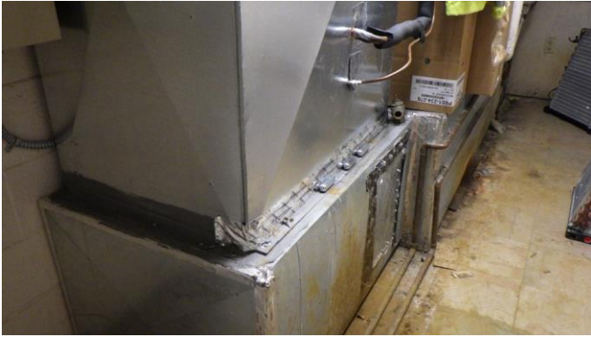
047065e 1/26/2023 Old built-in place air handler Mechanical room G137
