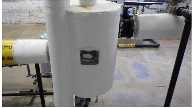
047031e 1/26/2023 HVAC distribution network hot water expansion tank TAN001 Mechanical room G520
