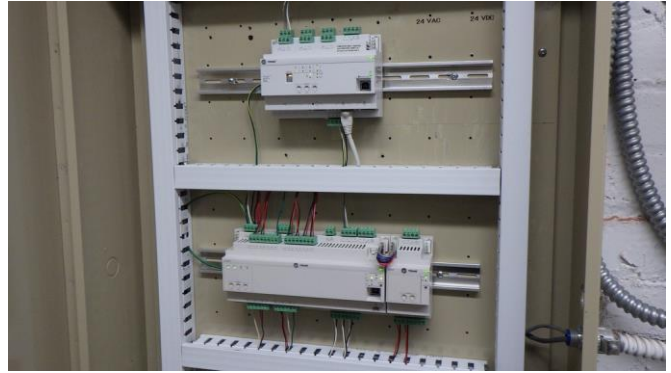
047037e 1/26/2023 HVAC DDC (Trane) controls panel Mechanical room G520
