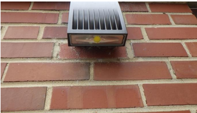
047079e 1/26/2023 LED wall pack exterior light fixture South exterior
