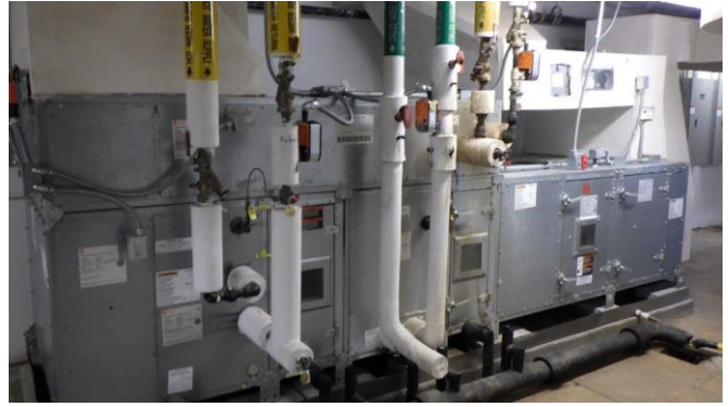
047040e 1/26/2023 Indoor AHU#1 Mechanical room G520
