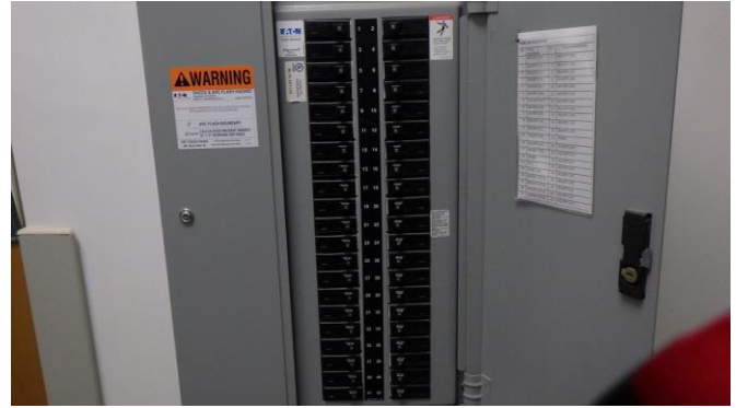
047010e 1/26/2023 Upgraded secondary electrical distribution panel R7 Office suite 2100
