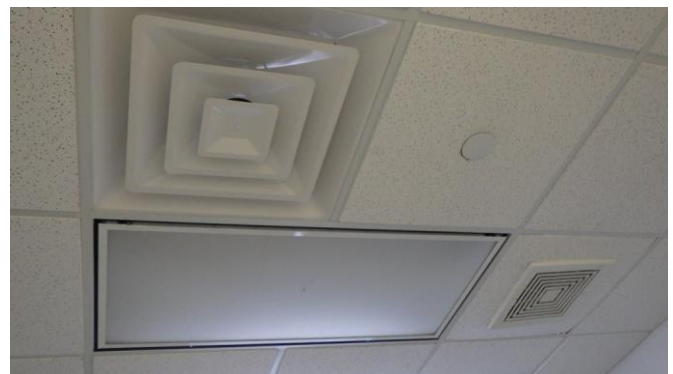
047006e 1/26/2023 Central HVAC air distribution supply grille, concealed fire suppression sprinkler head, toilet exhaust fan Men's restroom 2101
