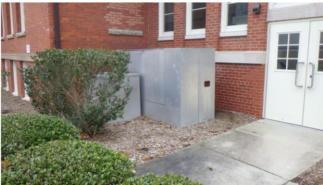
047085e 1/26/2023 Fire suppression system backflow preventer insulated box North exterior
