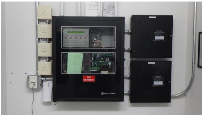
047055e 1/26/2023 Main fire alarm control panel FACP Electrical room G204
