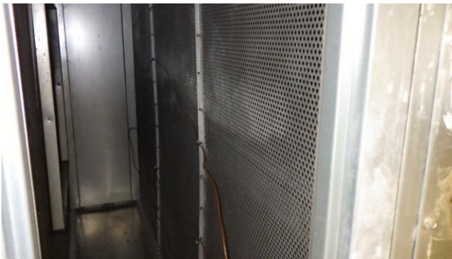
047063e 1/26/2023 AH#4 cooling coil section Mechanical room G301
