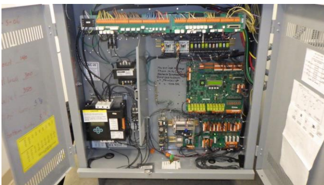
047057e 1/26/2023 Solid state elevator controller Elevator room G206
