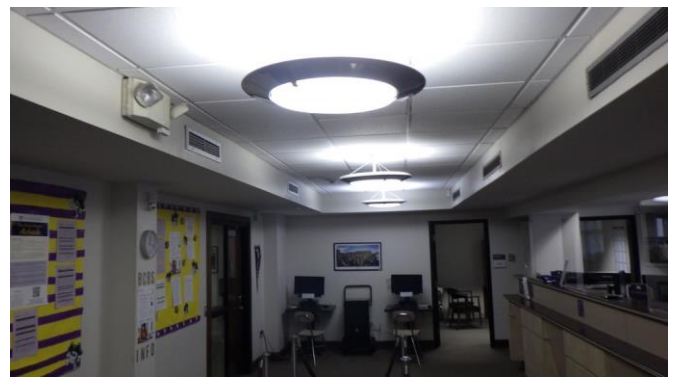
047074e 1/26/2023 Suspended LED interior light fixtures Office suite G120
