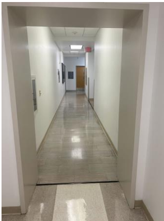
047011a 1/26/2023 Acoustical tile ceiling, vinyl floor tile (with and without asbestos), painted walls, wood doors Corridor
