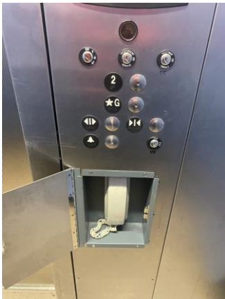
047014a 1/26/2023 Noncompliant elevator phone Elevator
