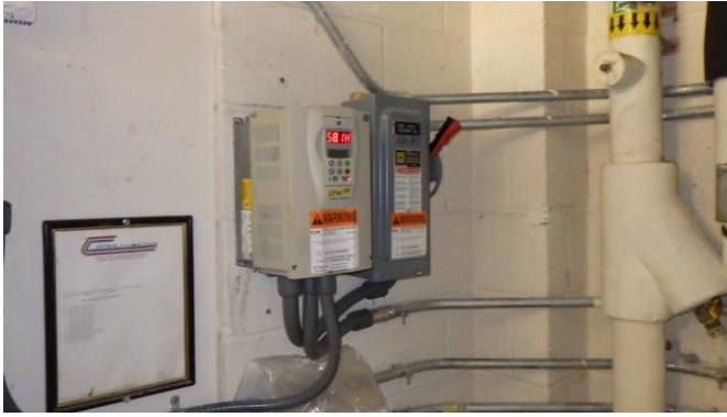
047071e 1/26/2023 AH#11 supply fan VFD, Square D Mechanical room G134
