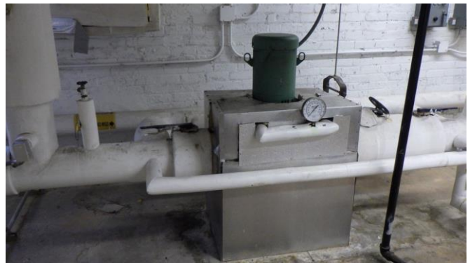
047041e 1/26/2023 HVAC distribution network chilled water pump 1 Mechanical room G520
