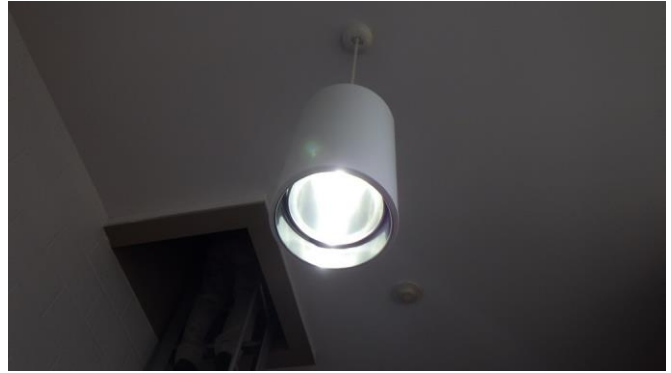
047007e 1/26/2023 Specialty interior light fixture Second floor, stair A
