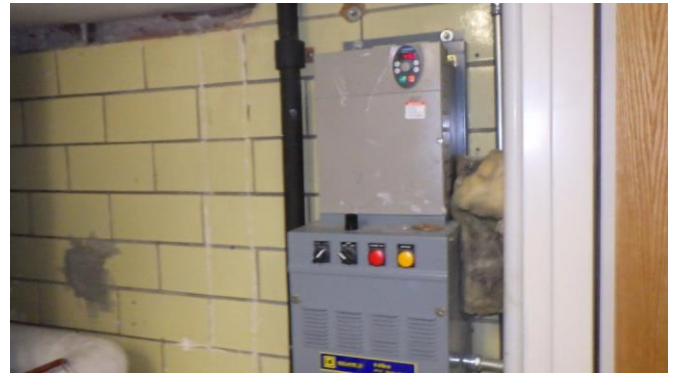
047060e 1/26/2023 AH#4 supply fan VFD, Square D Mechanical room G301
