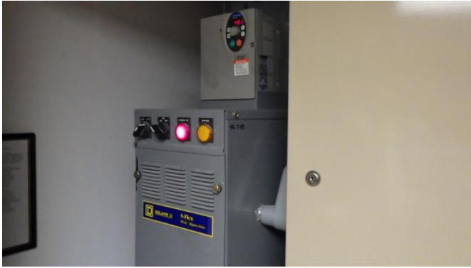
047053e 1/26/2023 AH supply fan VFD, Square D Mechanical room G410
