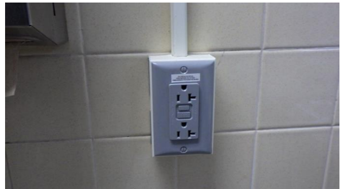
047005e 1/26/2023 GFCI electrical outlet Men's restroom 2101
