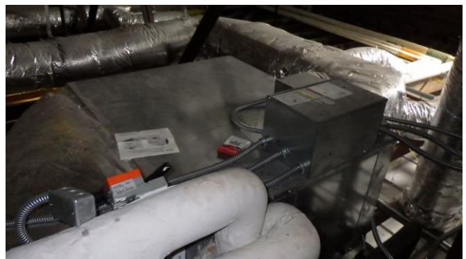
047021e 1/26/2023 FCU #3 Attic (above 2300)
