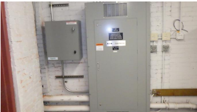
047087e 1/26/2023 Main electrical distribution panel MDP Electrical room G401
