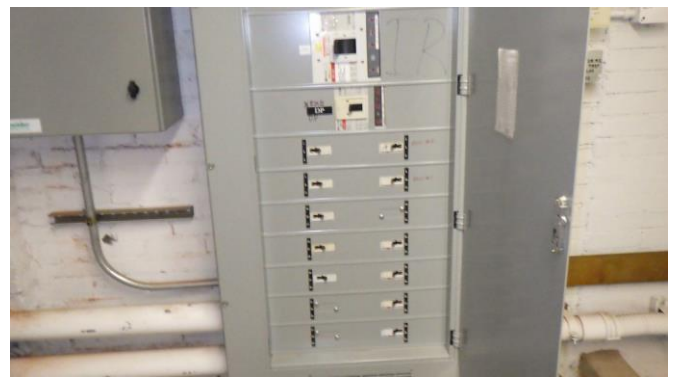
047088e 1/26/2023 Main electrical distribution panel MDP Electrical room G401
