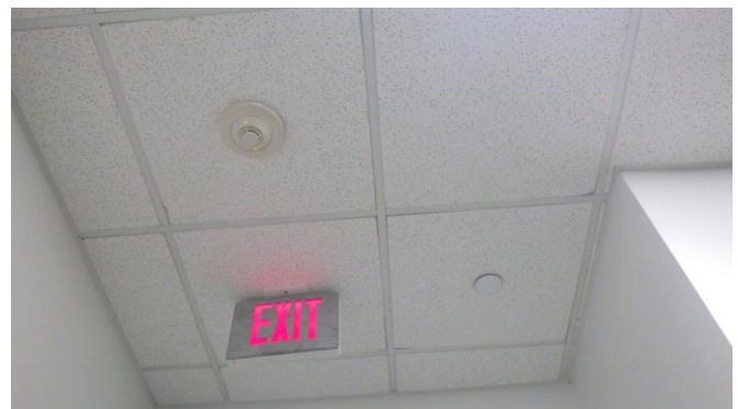
047012e 1/26/2023 Smoke/CO2 sensor, concealed fire suppression sprinkler head Office suite 2100
