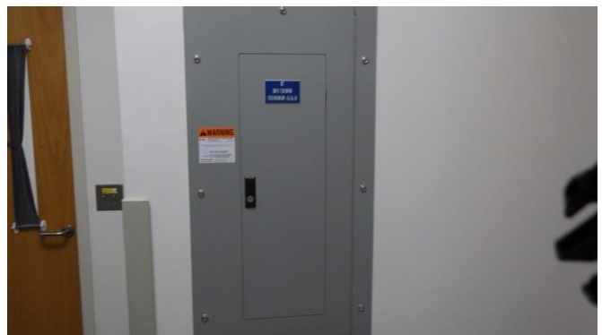
047009e 1/26/2023 Upgraded secondary electrical distribution panel R7 Office suite 2100
