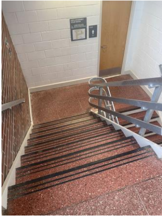
047004a 1/26/2023 CMU walls, terrazzo floor, noncompliant railing Stairwell
