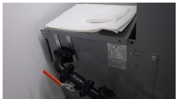
047058e 1/26/2023 Hydraulic passenger elevator #1 machine Elevator room G206
