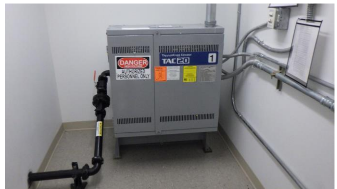
047056e 1/26/2023 Hydraulic passenger elevator #1 machine and controller Elevator room G206
