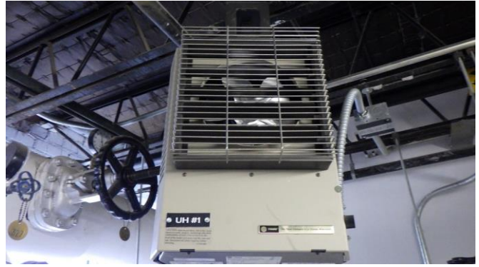
047025e 1/26/2023 Electric unit heater Mechanical room G520
