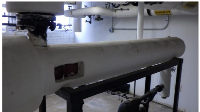
047029e 1/26/2023 Steam to hot water converter - shell-and-tube heat exchanger Mechanical room G520
