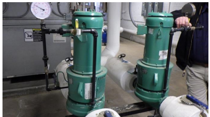
047033e 1/26/2023 HVAC distribution network heating hot water pumps 2, 3 Mechanical room G520
