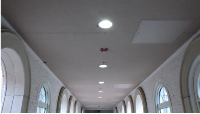
047083e 1/26/2023 Recessed CFL exterior light fixtures North side covered walk
