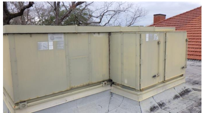
047002e 1/26/2023 Rooftop package unit RT#1 Roof, south side
