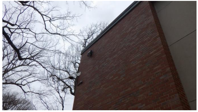
047078e 1/26/2023 LED wall pack exterior light fixture Southwest corner
