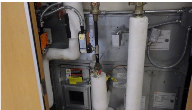
047051e 1/26/2023 HVAC distribution network chilled and heating hot water piping Mechanical room G403C
