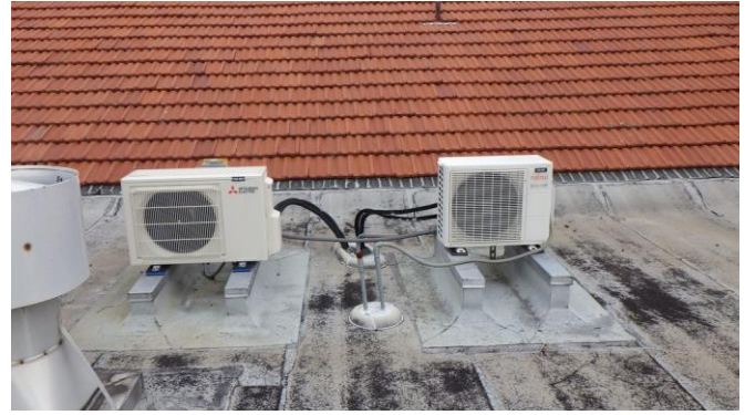
047001e 1/26/2023 Ductless split system condensing units CU#1, CU#2 Roof, south side
