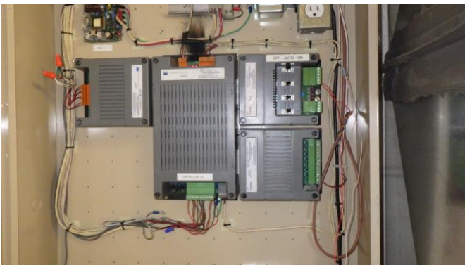
047067e 1/26/2023 HVAC controls panel Mechanical room G137
