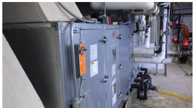
047042e 1/26/2023 Indoor AHU#2 Mechanical room G520
