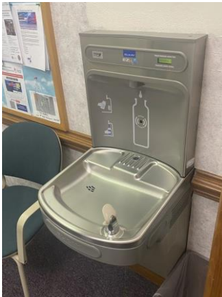
118014a 1/26/2023 Single-level water fountain Waiting room
