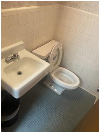
118001a 1/26/2023 Tile walls and floor, wall covering, lavatory, and tank water closet Restroom
