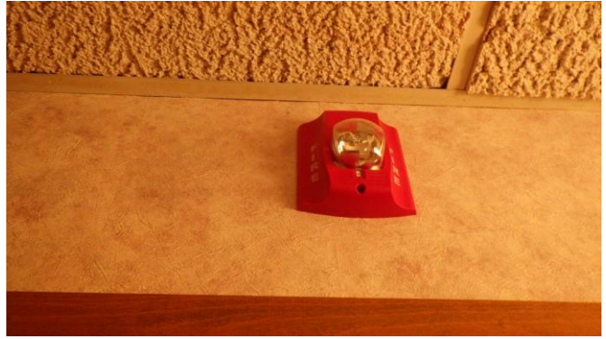
118010e 1/26/2023 Audible/visual alarm device Corridor
