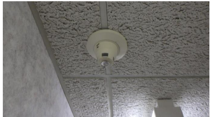
118014e 1/26/2023 Smoke alarm device Corridor
