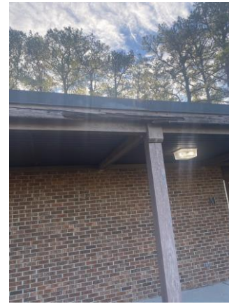
118025a 1/26/2023 Deteriorated roof awning Exterior
