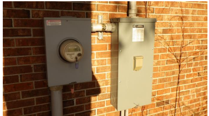
118008e 1/26/2023 Power meter Exterior wall
