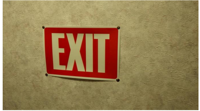
118013e 1/26/2023 Noncompliant exit sign Corridor
