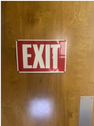
118008a 1/26/2023 Noncompliant exit signage Exit
