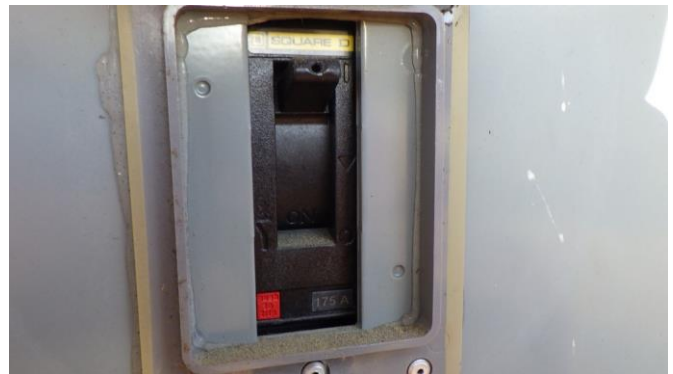
118009e 1/26/2023 Power distribution panel Main corridor
