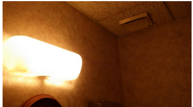
118002e 1/26/2023 Incandescent lighting Restroom
