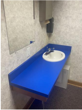
118013a 1/26/2023 Countertop lavatory Restroom
