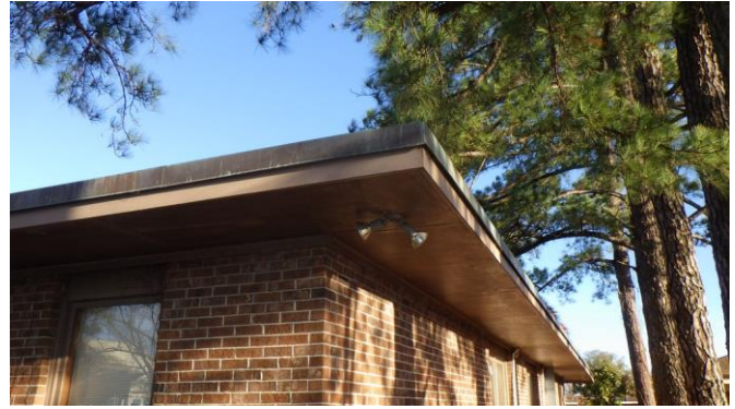
118004e 1/26/2023 Incandescent flood lighting Exterior corner soffit
