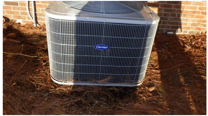
118007e 1/26/2023 Condensing unit 1 Site
