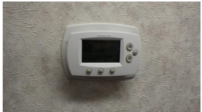
118006e 1/26/2023 Thermostat Hallway
