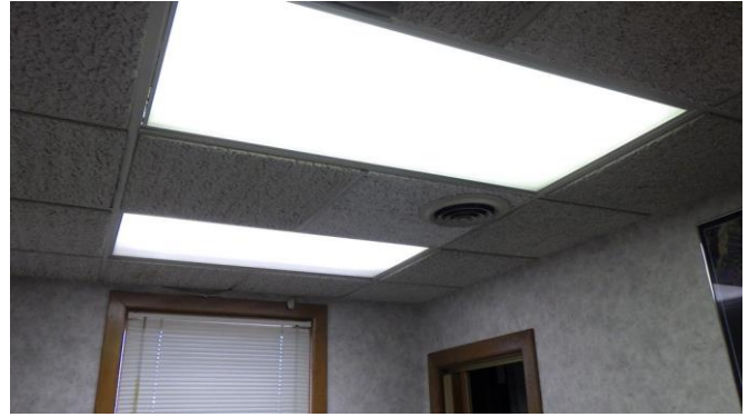
118001e 1/26/2023 T5 lay in troffers Commons area
