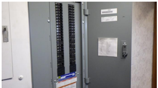
118012e 1/26/2023 Electrical distribution panel Corridor
