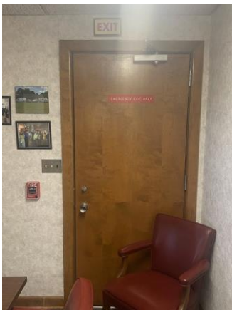
118012a 1/26/2023 Wood door with knob hardware and noncompliant exit sign Exit
