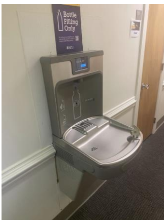
119006a 1/26/2023 Single-level water fountain Corridor
