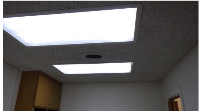
119001e 1/26/2023 T5 fluorescent lay-in troffer lighting Commons area
