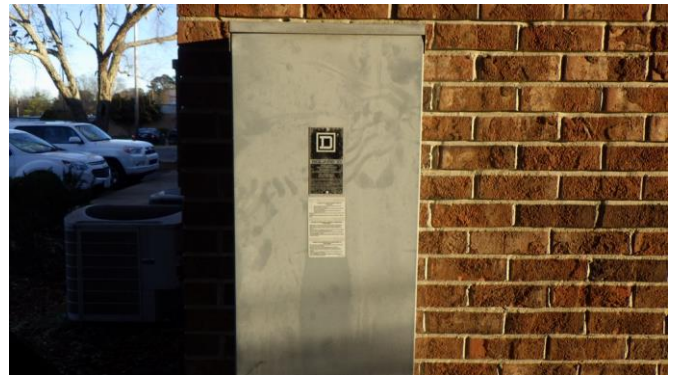
119011e 1/26/2023 Main electrical disconnect East exterior
