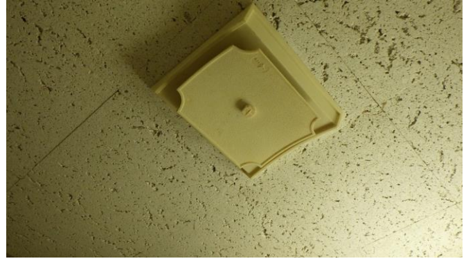
119013e 1/26/2023 Bathroom exhaust fan Bathroom
