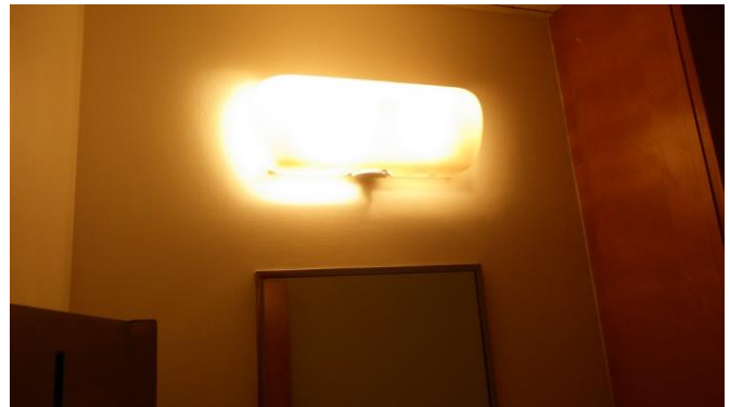
119002e 1/26/2023 Incandescent lighting Restroom
