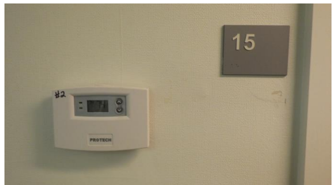
119009e 1/26/2023 Heat pump control thermostat Patient corridor
