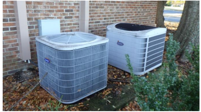
119010e 1/26/2023 Heat pump condensing units 1 and 2 East exterior
