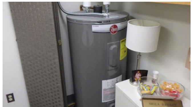
119006e 1/26/2023 Electric water heater 19611 Office 7
