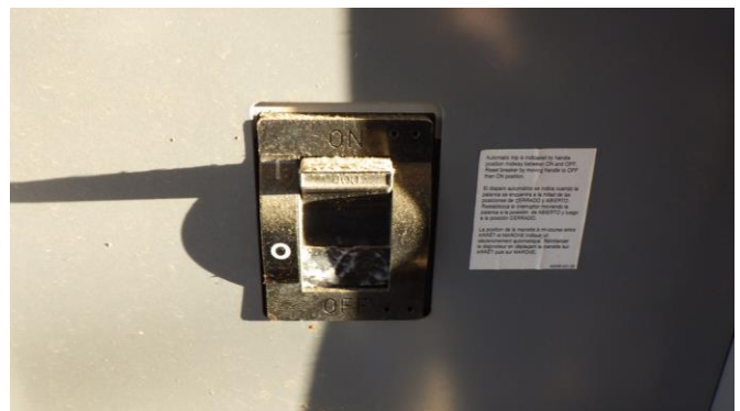
119012e 1/26/2023 Main electrical disconnect 400 amp breaker East exterior
