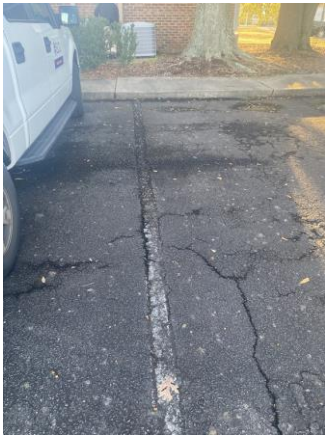
119020a 1/26/2023 Cracked asphalt parking lot Site
