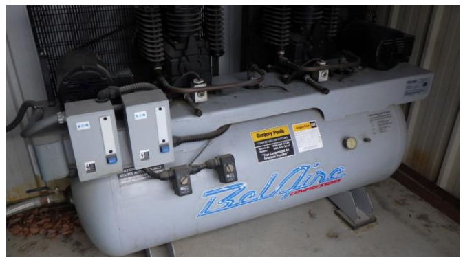
258021e 1/25/2023 Utility air compressor Electrical mechanical room
