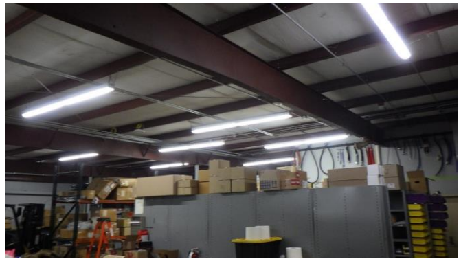
258002e 1/25/2023 Hi-bay fluorescent lighting Warehouse parts area
