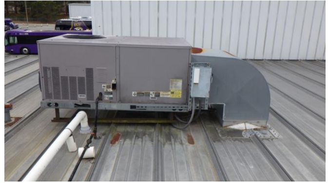
258019e 1/25/2023 Natural gas HVAC package unit Main roof
