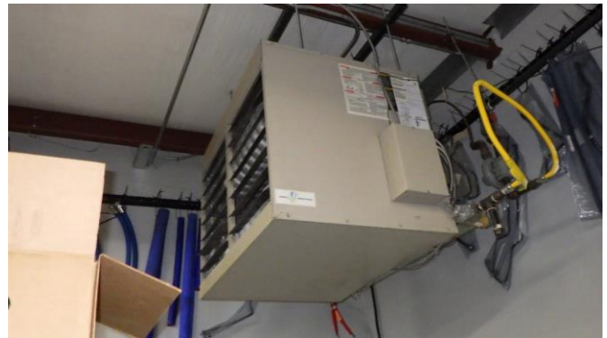
258020e 1/25/2023 Natural gas unit heater Warehouse parts area
