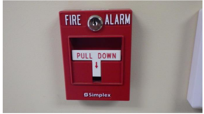
258007e 1/25/2023 Manual fire pull station Office area
