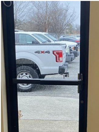
258017a 1/25/2023 Panic bar door hardware Secondary office exit
