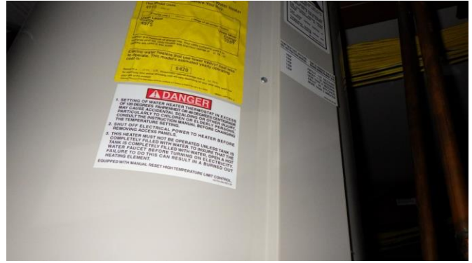
258022e 1/25/2023 Residential water heater Near 114
