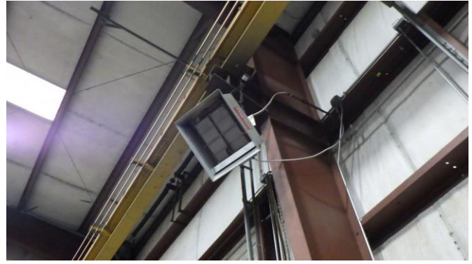
258016e 1/25/2023 Natural gas unit heater Wash bay
