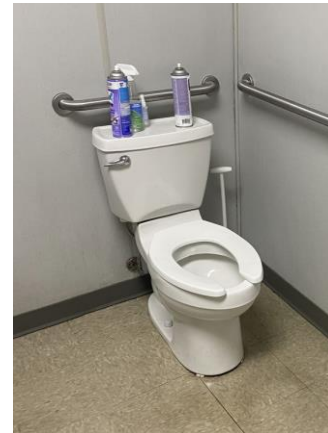
258024a 1/25/2023 Tank type water closet Restroom
