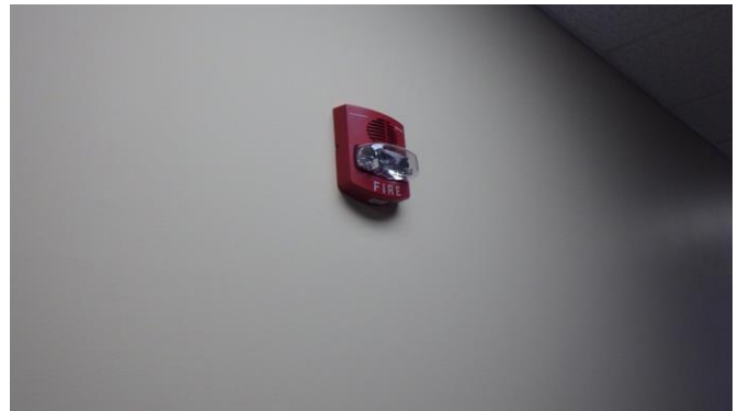
258008e 1/25/2023 Audio visual fire device Office area
