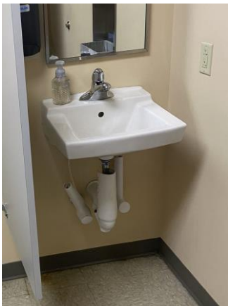
258025a 1/25/2023 Wall-hung lavatory Restroom
