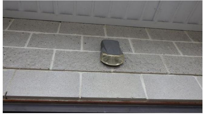
258004e 1/25/2023 LED exterior lighting Exterior wall
