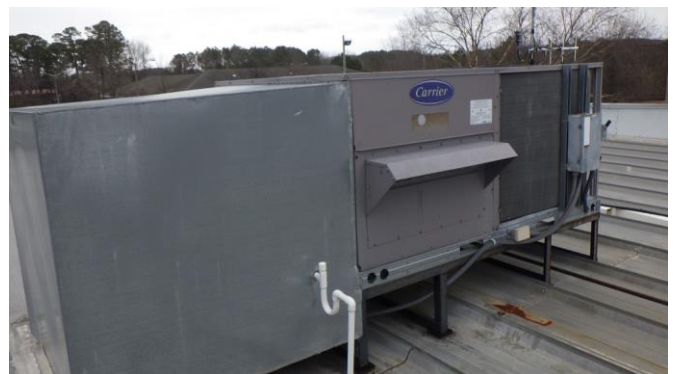
258018e 1/25/2023 Natural gas HVAC package unit Main roof
