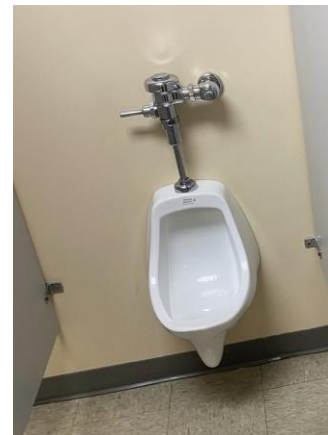
258026a 1/25/2023 Manual flush urinal Restroom
