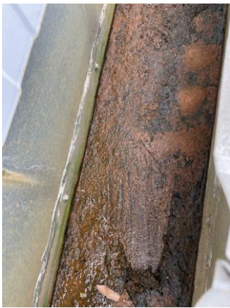
258003a 1/25/2023 Rusted rain gutter Office roof
