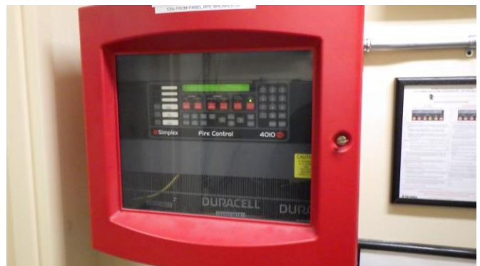
258006e 1/25/2023 Fire alarm panel Office area
