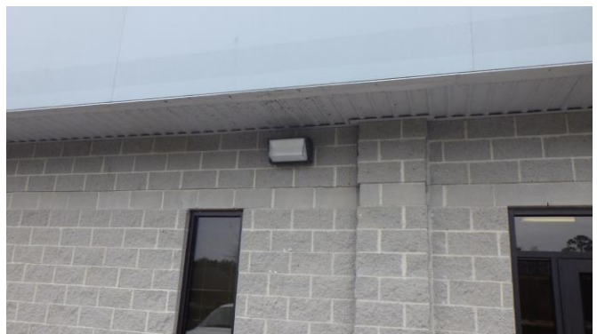
258003e 1/25/2023 HID exterior lighting Exterior wall
