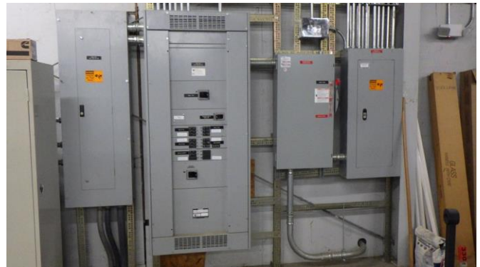
258005e 1/25/2023 Main electrical disconnects Electrical mechanical room
