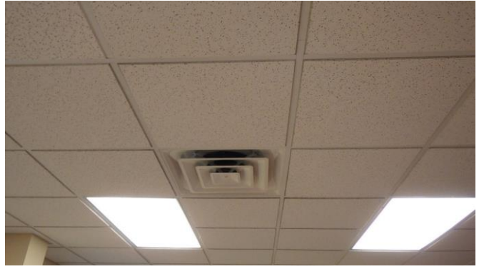
258001e 1/25/2023 Fluorescent indoor lighting Office area
