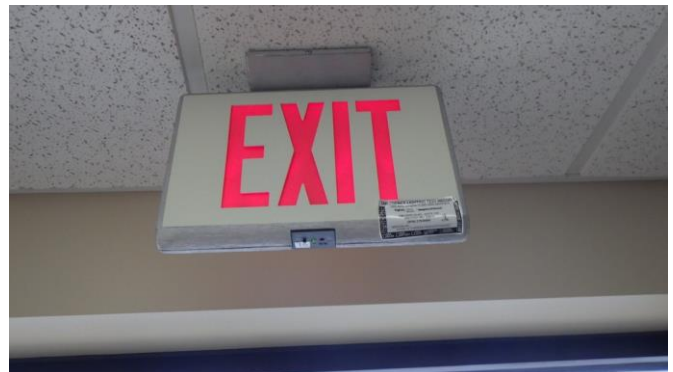
258009e 1/25/2023 Illuminated exit sign Office area
