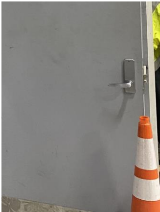
258014a 1/25/2023 Lever style door hardware Office to wash bay
