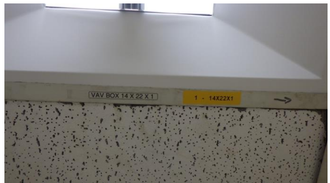
097030e 1/25/2023 VAV box label Men's restroom 337
