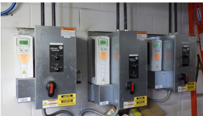
097052e 1/25/2023 VFDs for AHU-1 RF, SF, and HHWP Mechanical 02
