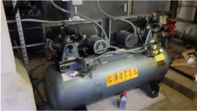
097048e 1/25/2023 HVAC controls air compressor Mechanical 02
