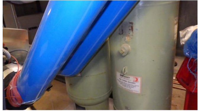
097043e 1/25/2023 Original HVAC storage tanks Mechanical 02
