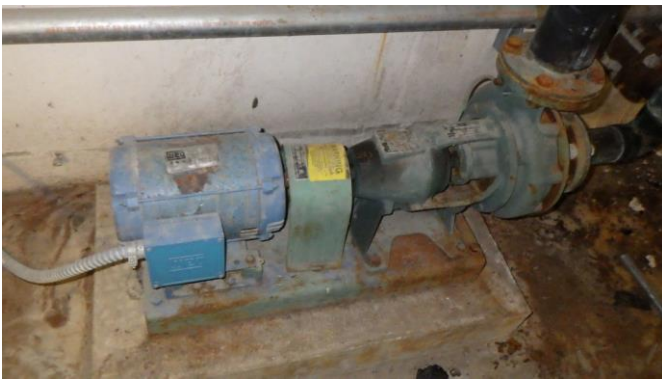
097050e 1/25/2023 Abandoned domestic water pump Mechanical 02
