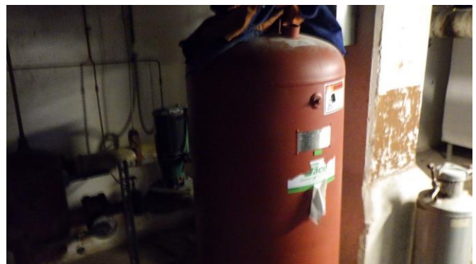
097042e 1/25/2023 HVAC expansion tank Mechanical 02
