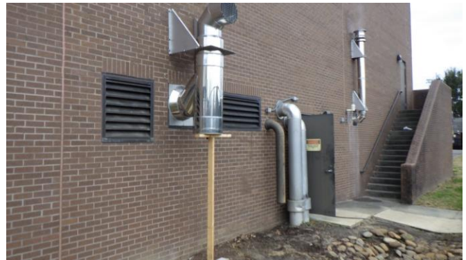
097038e 1/25/2023 New boiler exhaust and original central plant utility entrances West elevation, mechanical basement
