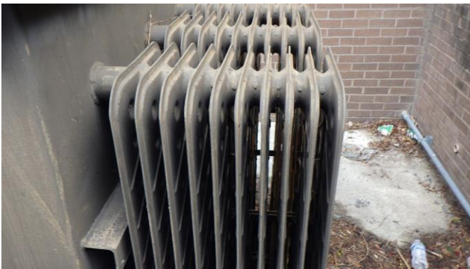
097062e 1/25/2023 Primary electrical transformer cooling fins South elevation
