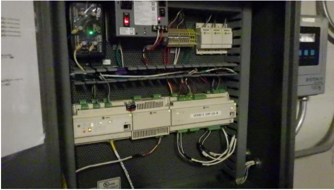
097054e 1/25/2023 CHW pump VFDs Mechanical 02
