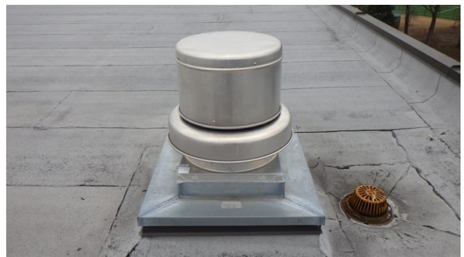
097006e 1/25/2023 Roof exhauster EF-2 Roof
