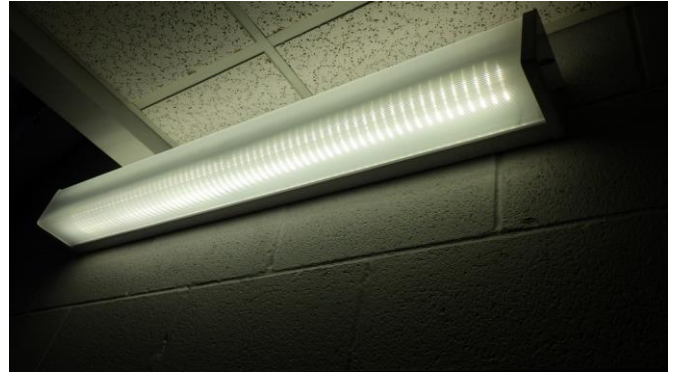
097010e 1/25/2023 Surface-mounted interior light fixture Stair 326
