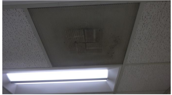
097028e 1/25/2023 Central HVAC distribution grill Men's restroom 337
