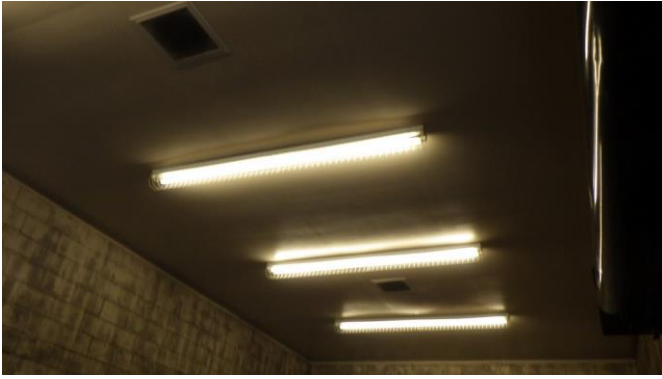
097072e 1/25/2023 Surface mounted interior light fixture South elevation, lawn maintenance building
