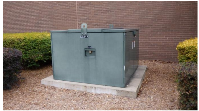
097075e 1/25/2023 Primary electrical distribution network high voltage switch East elevation
