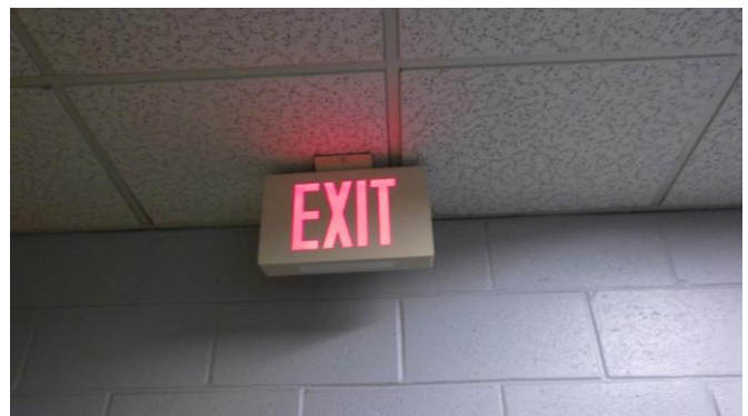
097012e 1/25/2023 Illuminated emergency exit sign Hall 330
