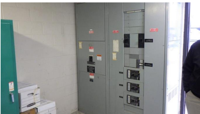
097064e 1/25/2023 Main electrical distribution switchboard Electrical 03
