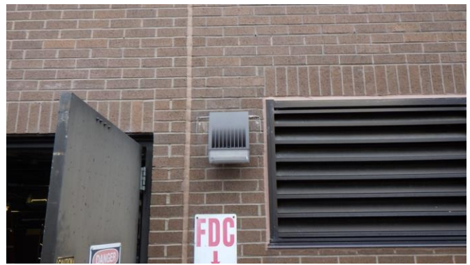
097063e 1/25/2023 LED exterior wall pack light fixture South elevation
