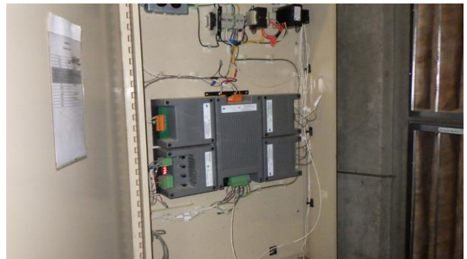
097024e 1/25/2023 HVAC DDC control panel Mechanical 334
