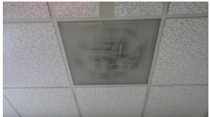
097015e 1/25/2023 Central HVAC return air grill Hall 330
