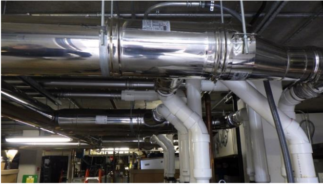
097060e 1/25/2023 Domestic water boiler exhaust network Mechanical 02
