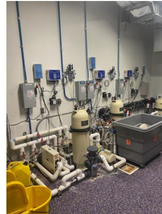
097002e 1/25/2023 Spa pool equipment Pump room 134
