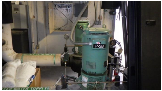
097055e 1/25/2023 HVAC DDC control panel Mechanical 02
