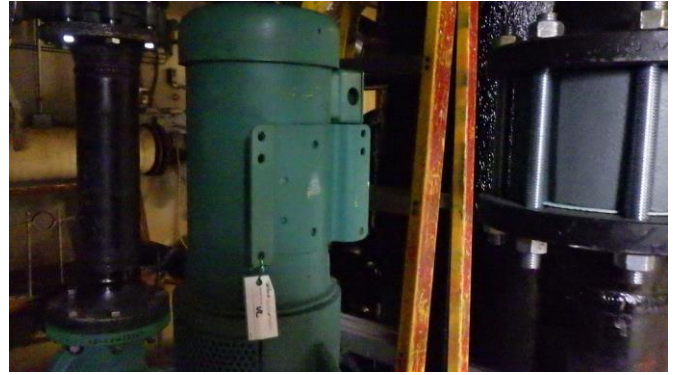
097040e 1/25/2023 Heating hot water electric motor driven pump Mechanical 02
