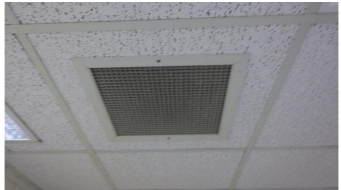
097029e 1/25/2023 Central HVAC return air grill Men's restroom 337
