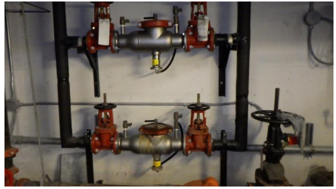
097049e 1/25/2023 Domestic water backflow preventers Mechanical 02
