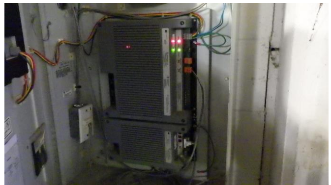
097057e 1/25/2023 HVAC controls panel (older generation) Mechanical 02
