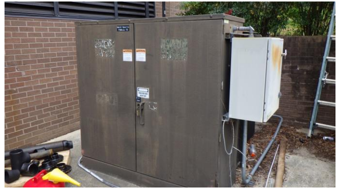
097061e 1/25/2023 Primary electrical transformer South elevation
