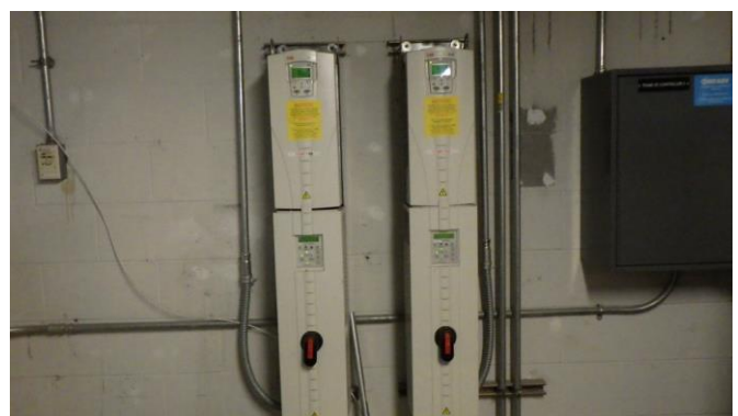
097053e 1/25/2023 HHW pump VFDs 2B and 3A Mechanical 02
