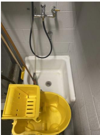
097015a 1/24/2023 Cast-iron utility sink Custodial closet
