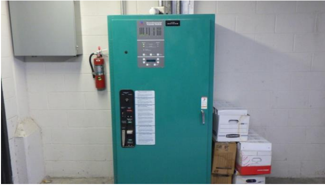
097066e 1/25/2023 Emergency power ATS#2 Electrical 03
