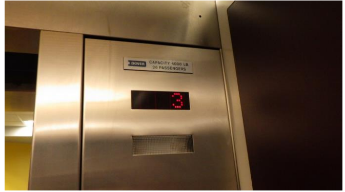
097004e 1/25/2023 Elevator identification placard Elevator A cab
