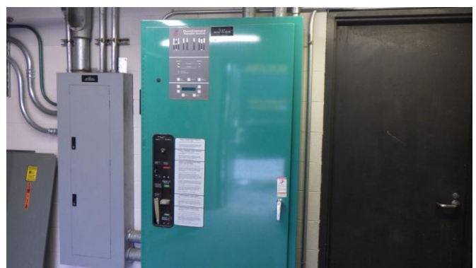
097065e 1/25/2023 Emergency power ATS#1 Electrical 03
