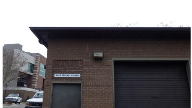
097071e 1/25/2023 HID exterior wall pack light fixture South elevation, lawn maintenance building
