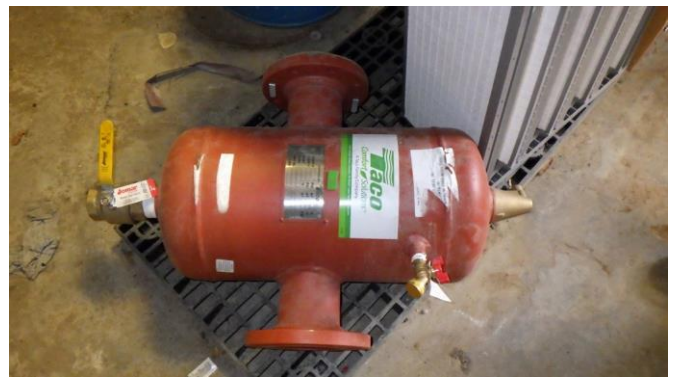
097051e 1/25/2023 New HVAC expansion tank Mechanical 02
