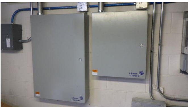
097058e 1/25/2023 HVAC DDC control panel (older generation) Mechanical 02
