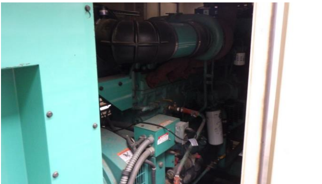
097068e 1/25/2023 Diesel fuel emergency power generator South elevation, emergency generator building
