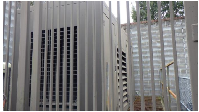
097067e 1/25/2023 Diesel fuel emergency power generator South elevation, emergency generator building
