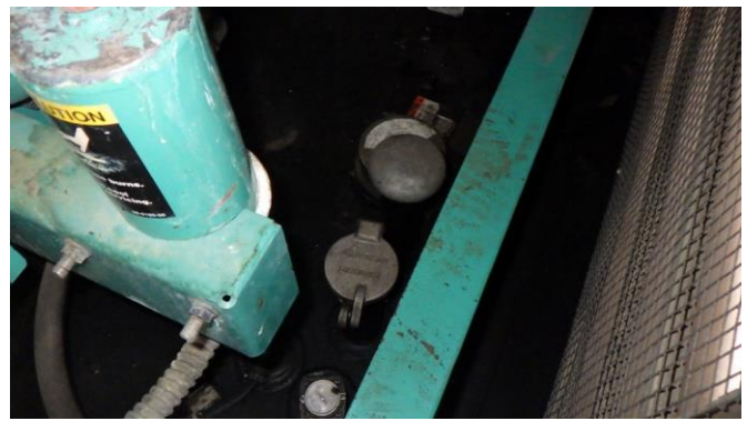
097069e 1/25/2023 Diesel fuel day tank under emergency generator South elevation, emergency generator building
