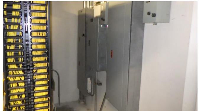
097032e 1/25/2023 Secondary electrical distribution panels Electrical 340
