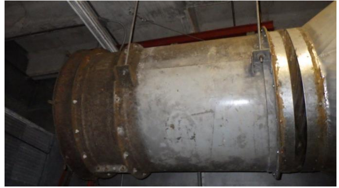
097016e 1/25/2023 Air handler AHU-1 supply fan Mechanical 334
