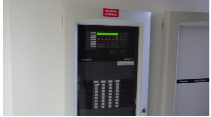
097037e 1/25/2023 Main fire alarm control panel Lobby 101
