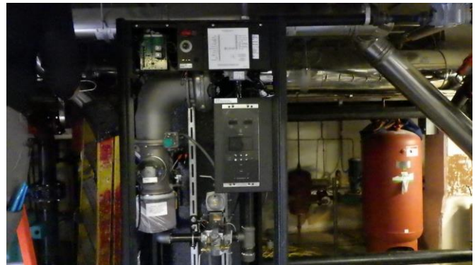
097041e 1/25/2023 New high efficiency natural gas heating hot water boiler Mechanical 02
