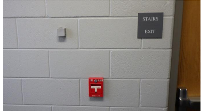
097031e 1/25/2023 Manual pull station Hall 333
