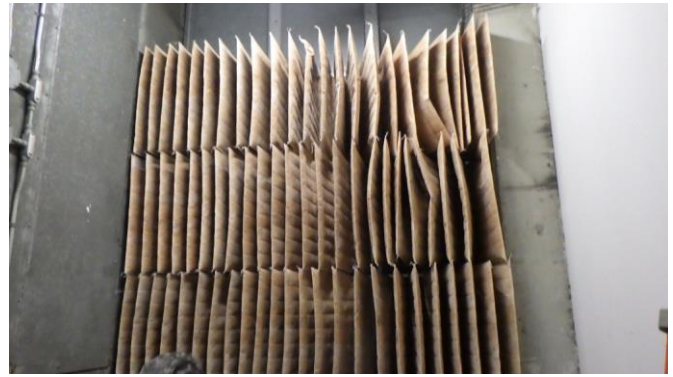
097025e 1/25/2023 AHU-1 filter section Mechanical 334
