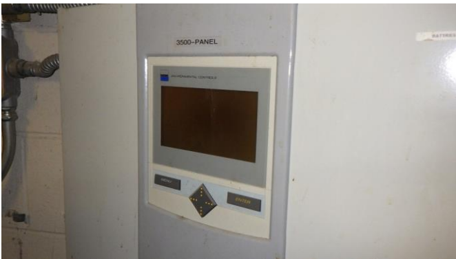
097056e 1/25/2023 Chilled water pumps 2A and 2B Mechanical 02
