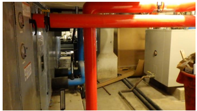
097045e 1/25/2023 Hot water and chiller water piping to AHU -1 coil sections Mechanical 02
