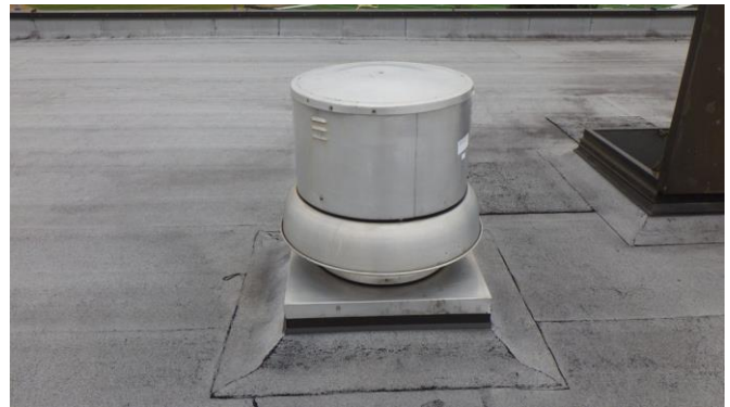
097008e 1/25/2023 Powered roof exhauster Roof
