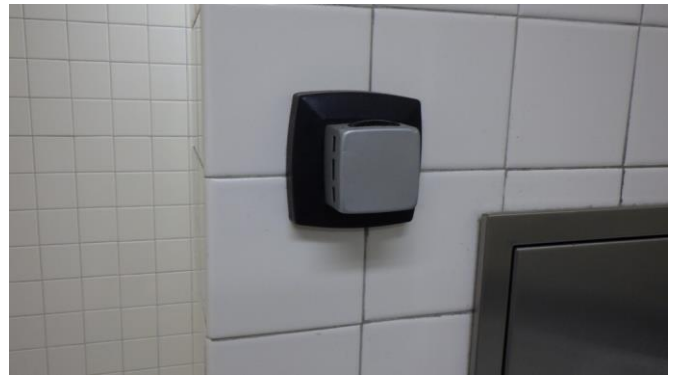
097026e 1/25/2023 Original temperature sensor/thermostat Men's restroom 337
