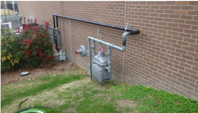
097074e 1/25/2023 Natural gas supply meter South elevation
