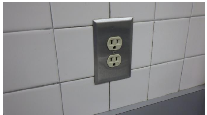
097027e 1/25/2023 Normal electrical outlet (no GFCI) Men's restroom 337
