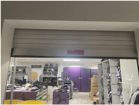
097035a 1/24/2023 Overhead roll up window Equipment room
