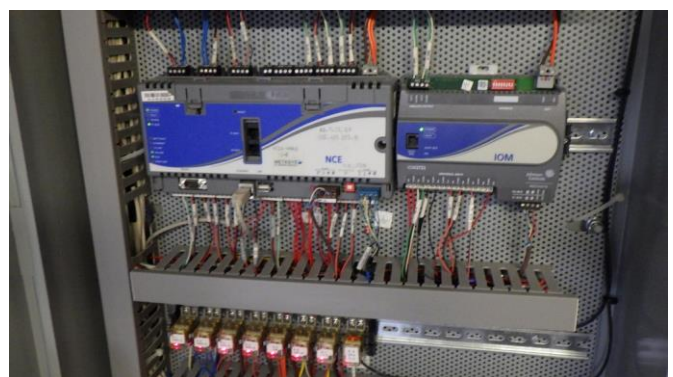
097059e 1/25/2023 HVAC DDC control panels Mechanical 02
