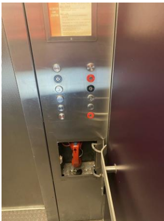
097021a 1/24/2023 Noncompliant phone in elevator panel Elevator
