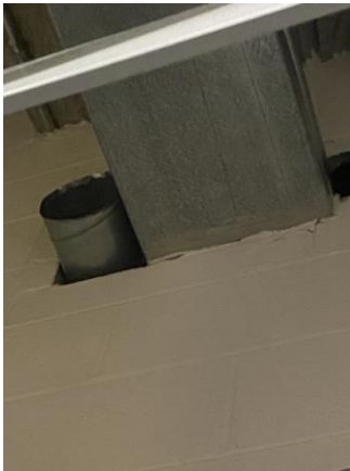
097016a 1/24/2023 Unsealed penetrations Mechanical closet
