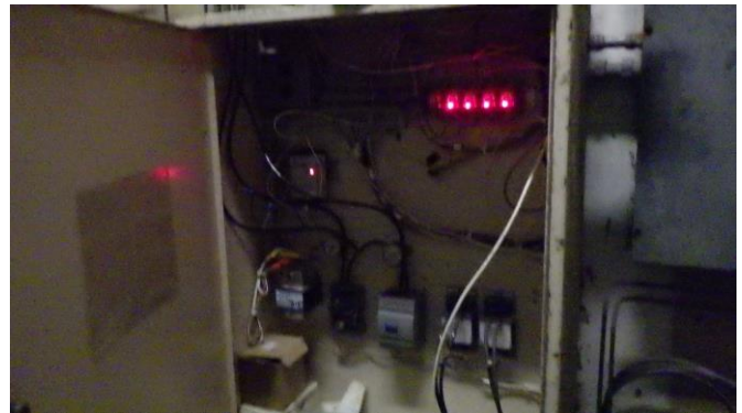
097023e 1/25/2023 HVAC pneumatics control panel Mechanical 334
