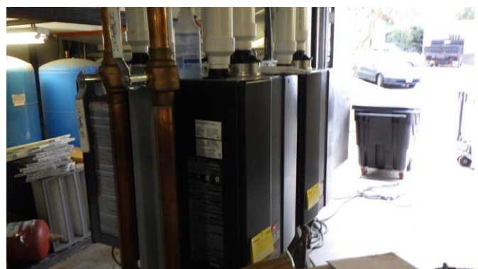
097047e 1/25/2023 New tankless domestic hot water heater rack (4 units) Mechanical 02
