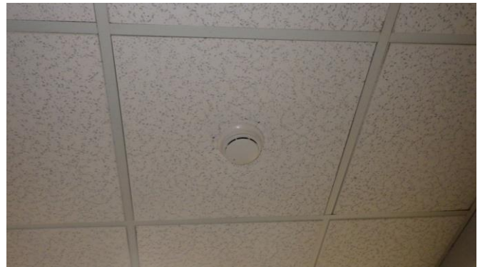
097014e 1/25/2023 Smoke/CO2 sensor Hall 330
