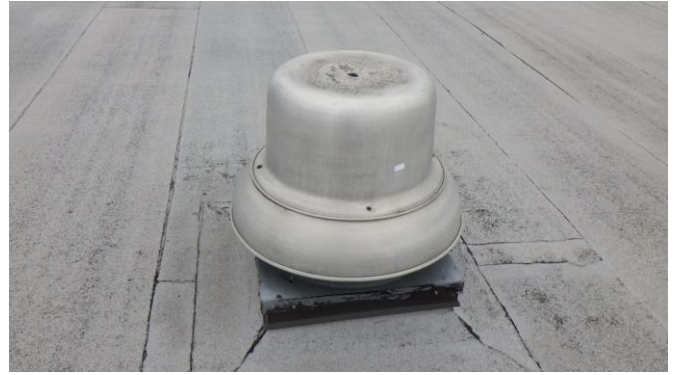
097007e 1/25/2023 Powered roof exhauster Roof
