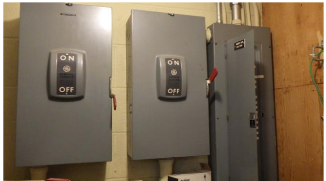
098015e 1/25/2023 Main electrical disconnects Electrical room
