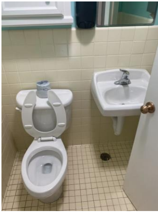
098013a 1/25/2023 Tile walls and floor, ACT, tank water closet, and wall-hung lavatory Restroom
