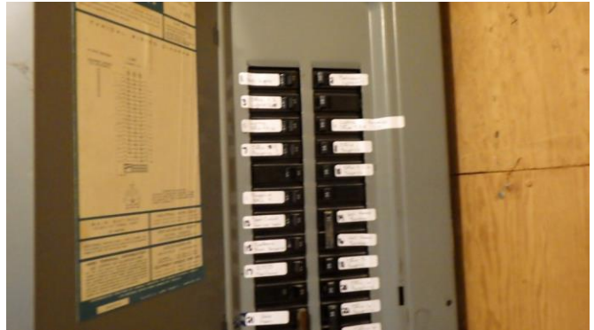
098014e 1/25/2023 Electrical distribution panel Electrical room
