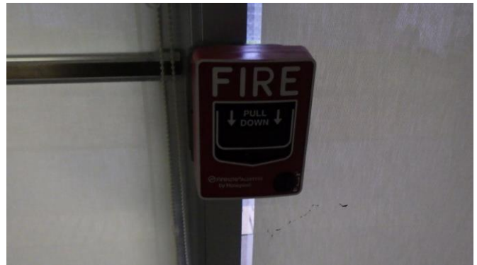
098008e 1/25/2023 Manual alarm pull station Rear exit door
