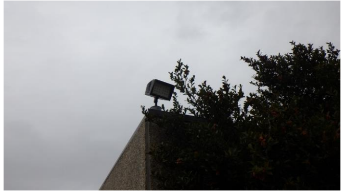
098004e 1/25/2023 HID area lighting Roof gable
