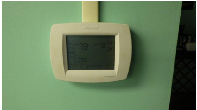
098011e 1/25/2023 HVAC thermostat Main corridor
