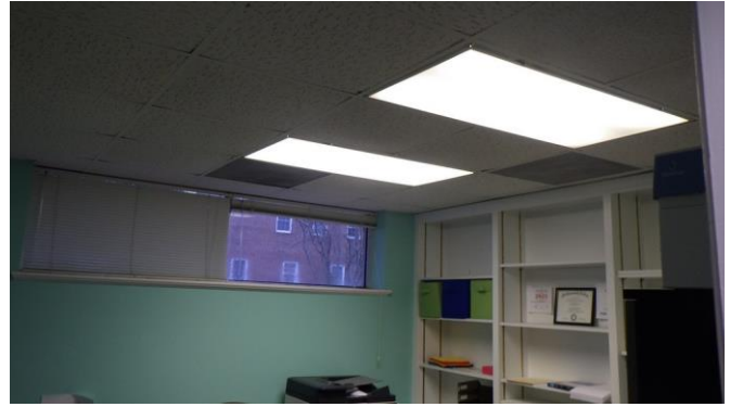
098001e 1/25/2023 Fluorescent troffer lights Office area
