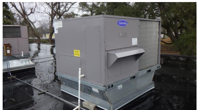
098009e 1/25/2023 Natural gas package unit Main room
