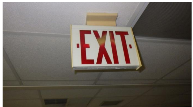
098003e 1/25/2023 Illuminated exit lighting Main corridor
