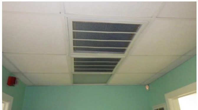
098012e 1/25/2023 HVAC distribution vent Office
