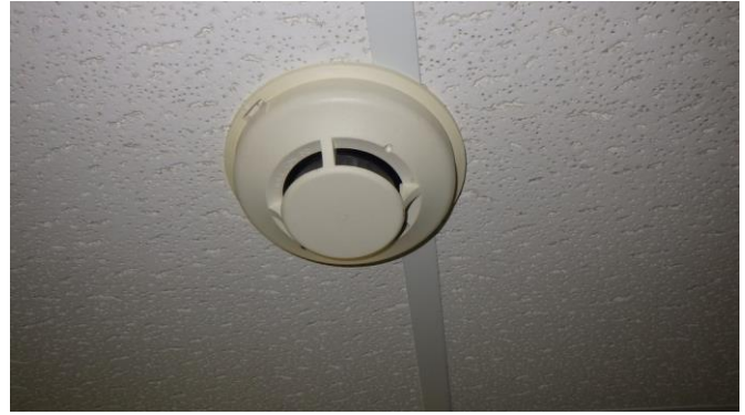
098007e 1/25/2023 Smoke detector Office ceiling
