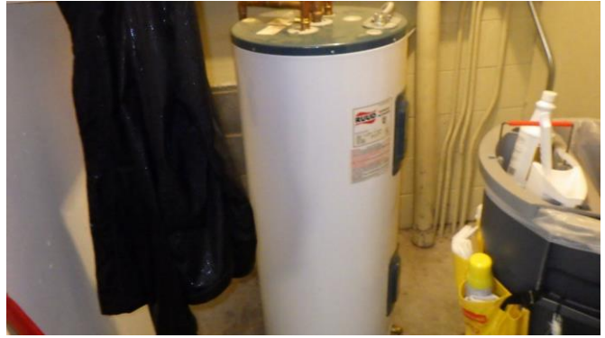
098013e 1/25/2023 Residential electric water heater Mechanical room
