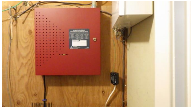
098005e 1/25/2023 Fire alarm power panel Electrical room
