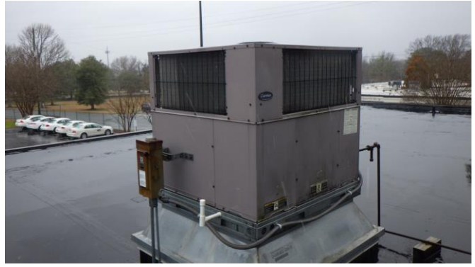
098010e 1/25/2023 Natural gas package unit Main room
