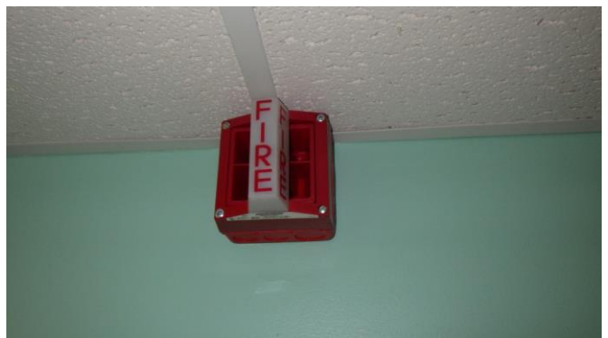
098006e 1/25/2023 Audio visual alarm device Restroom wall
