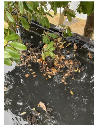
098021a 1/25/2023 Black EPDM roof and clogged drain Roof
