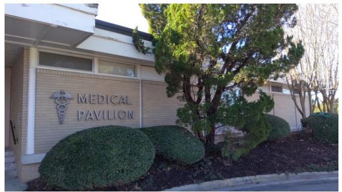
099034a 1/26/2023 Brick exterior, glazing, weathered fascia board Exterior
