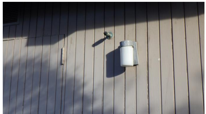
099003e 1/26/2023 Incandescent exterior sconce light Exterior wall
