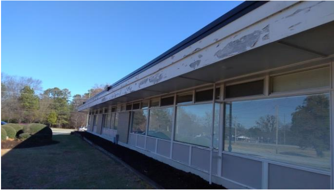
099035a 1/26/2023 Brick exterior, glazing, weathered fascia board Exterior
