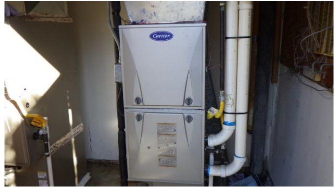
099016e 1/26/2023 HVAC indoor fan unit Suite mechanical room
