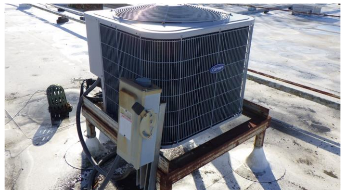
099012e 1/26/2023 HVAC condensing unit Main roof
