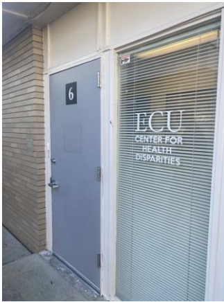
099011a 1/26/2023 Hollow metal door with lever hardware Exterior door
