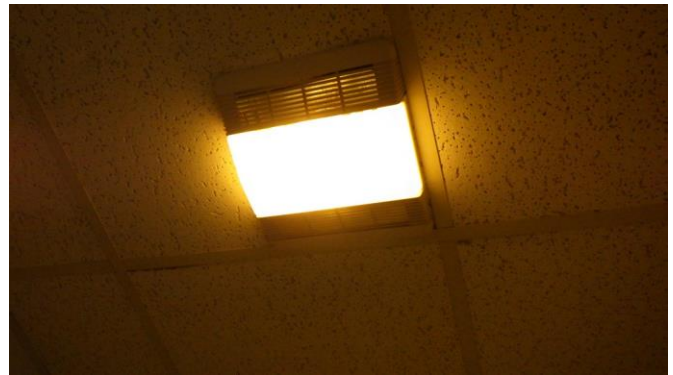
099002e 1/26/2023 Incandescent lighting Exterior soffit
