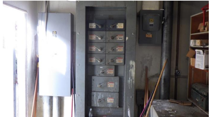
099005e 1/26/2023 Main switchgear panel Main electrical room
