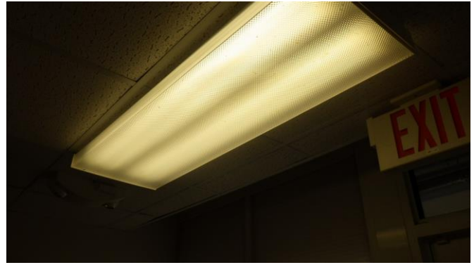
099001e 1/26/2023 Fluorescent lighting General office area
