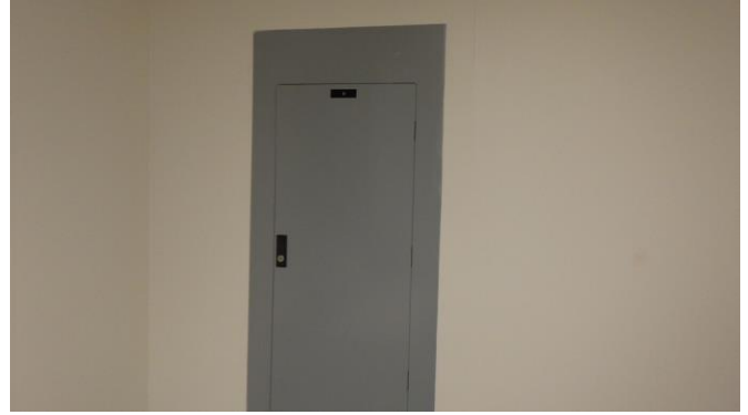
099004e 1/26/2023 120 volt electrical distribution Suite electrical room
