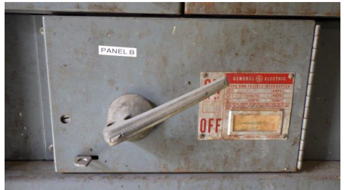
099006e 1/26/2023 Main switchgear disconnect Main electrical room
