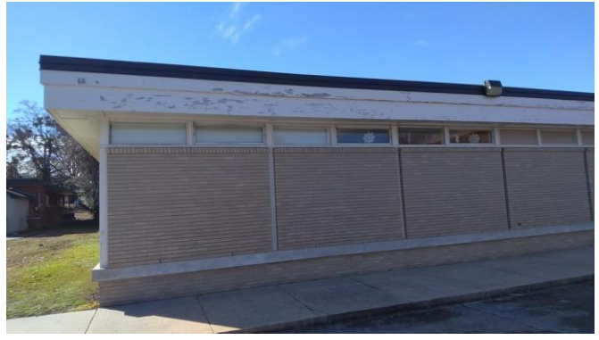
099036a 1/26/2023 Brick exterior, glazing, weathered fascia board Exterior
