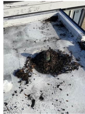
099028a 1/26/2023 EPDM roof, clogged drain Roof
