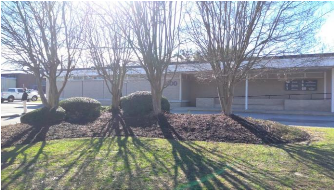
099037a 1/26/2023 Brick exterior, glazing, weathered fascia board Exterior
