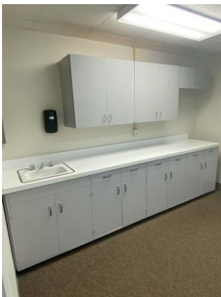
099006a 1/26/2023 Acoustical tile ceiling, carpet, painted walls, casework with a sink Break room
