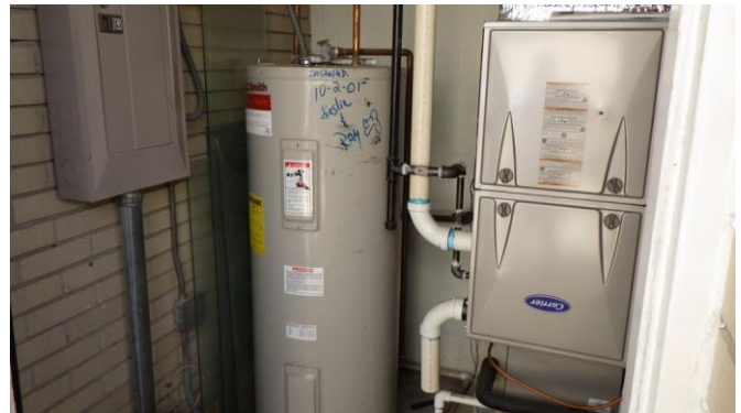
099017e 1/26/2023 Commercial gas water heater Suite mechanical room
