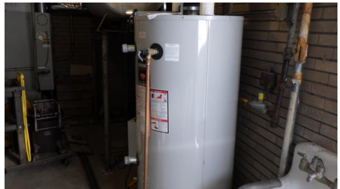
099018e 1/26/2023 Residential electric water heater Suite mechanical room
