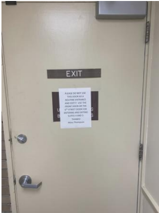
099010a 1/26/2023 Painted hollow metal door with noncompliant exit sign Corridor
