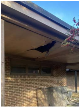
117020a 1/26/2023 Damage to roof system Front soffit area
