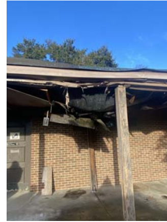
117019a 1/26/2023 Damage to roof system Front soffit area
