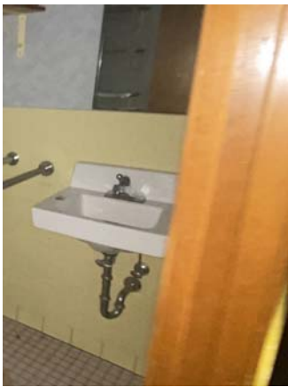
117016a 1/26/2023 Wall-hung lavatory Restroom
