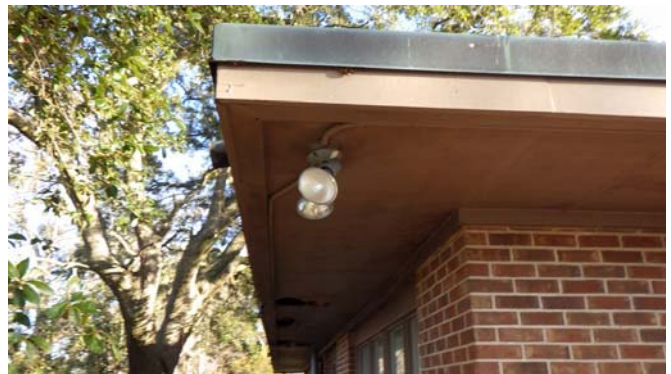
117003e 1/26/2023 Incandescent flood lighting Corner soffit
