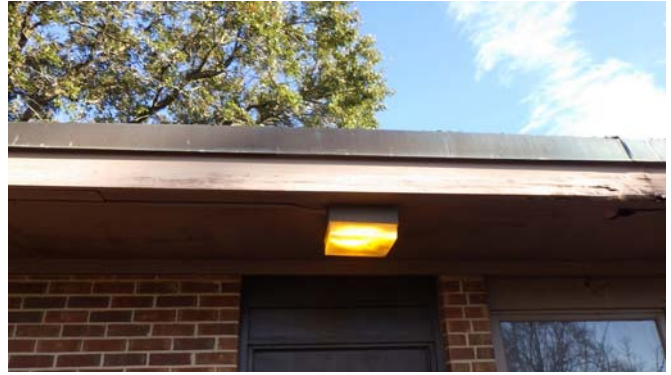
117004e 1/26/2023 Incandescent surface mount light Building entrance
