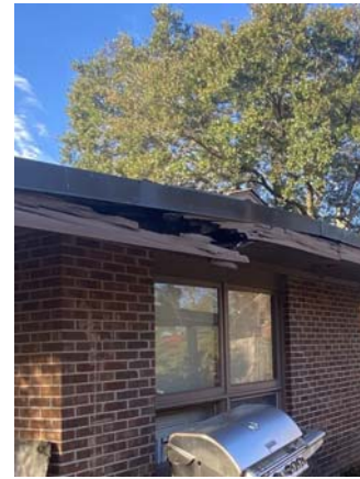
117021a 1/26/2023 Damage to roof system East elevation
