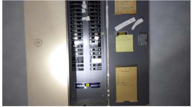
117010e 1/26/2023 Electrical distribution panel Mechanical area
