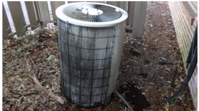
117008e 1/26/2023 Heat pump condensing units 2 East elevation
