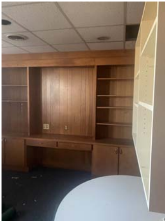
117005a 1/26/2023 Suspended acoustical ceiling Office area
