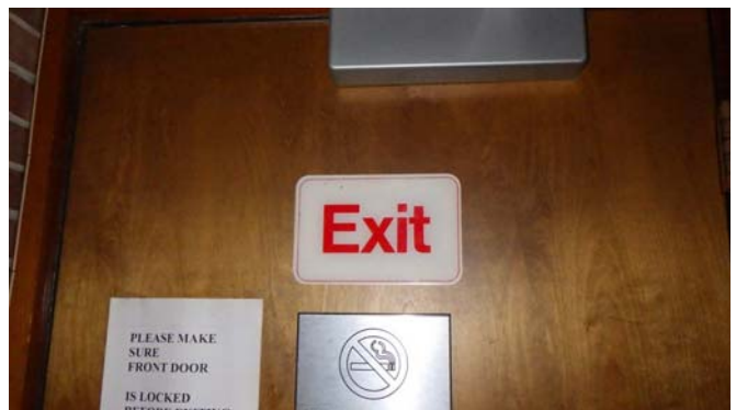
117012e 1/26/2023 Noncompliant exit sign Corridor area
