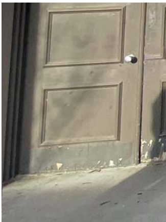
117012a 1/26/2023 Noncompliant knob hardware Main entrance
