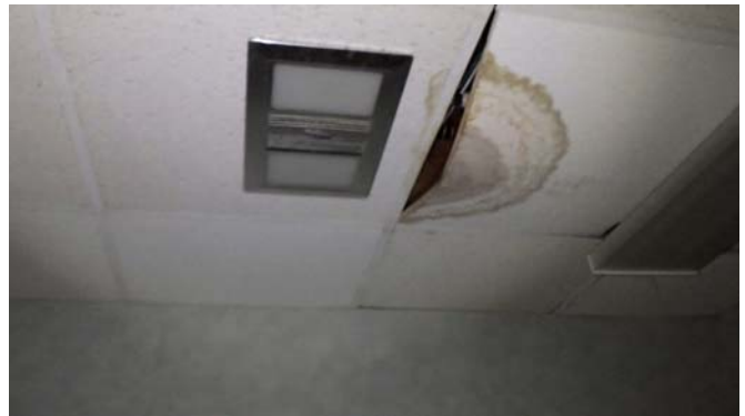
117002e 1/26/2023 Recessed lighting Corridor
