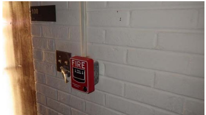
117011e 1/26/2023 Manual fire alarm device Corridor at exit
