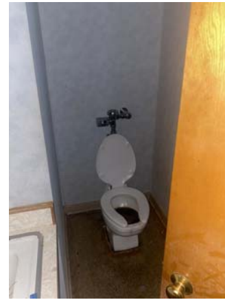
117015a 1/26/2023 Tankless water closet Restroom
