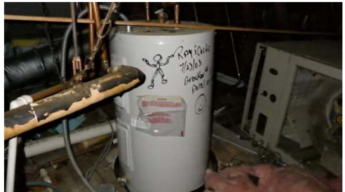
117005e 1/26/2023 Electric water heater 19602 Attic space
