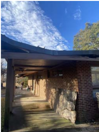
117002a 1/26/2023 Damage to roof system Front breezeway
