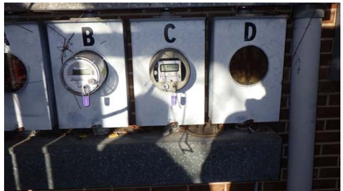
117009e 1/26/2023 Main electrical meter base East elevation
