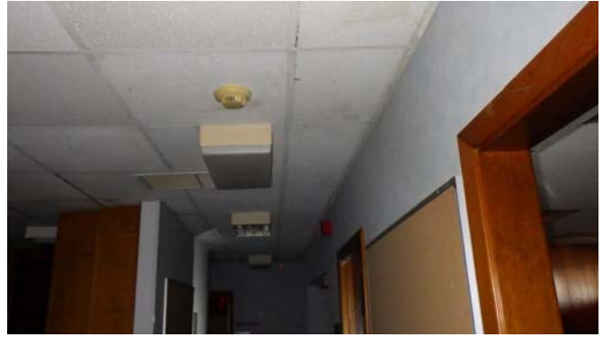
117001e 1/26/2023 Incandescent lighting Commons area
