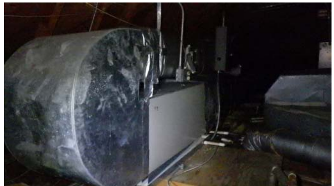
117006e 1/26/2023 Indoor fan unit 1 Attic space
