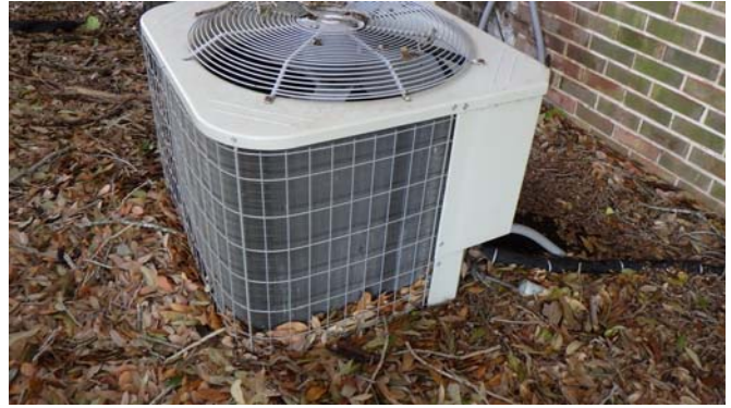
117007e 1/26/2023 Heat pump condensing units 1 East elevation
